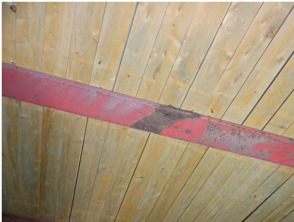
Photo 20: Beam 2B, span 2 near pier 2, looking west - the bottom flange cover plate has an area of heavy rust with minor section loss.
