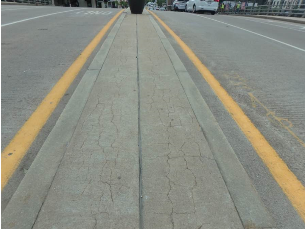
Photo 3: Typical numerous hairline map cracks throughout the median
