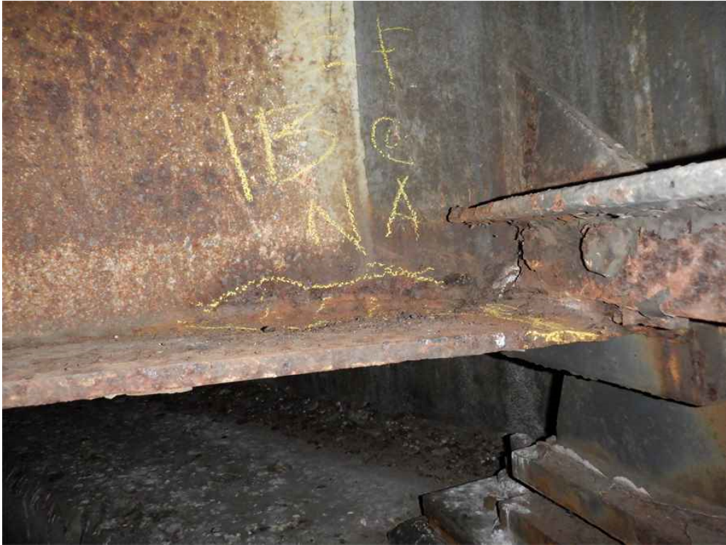
Photo 7: Beam 1B, span 1, at north abutment, looking northwest - section loss at east side bottom flange.
