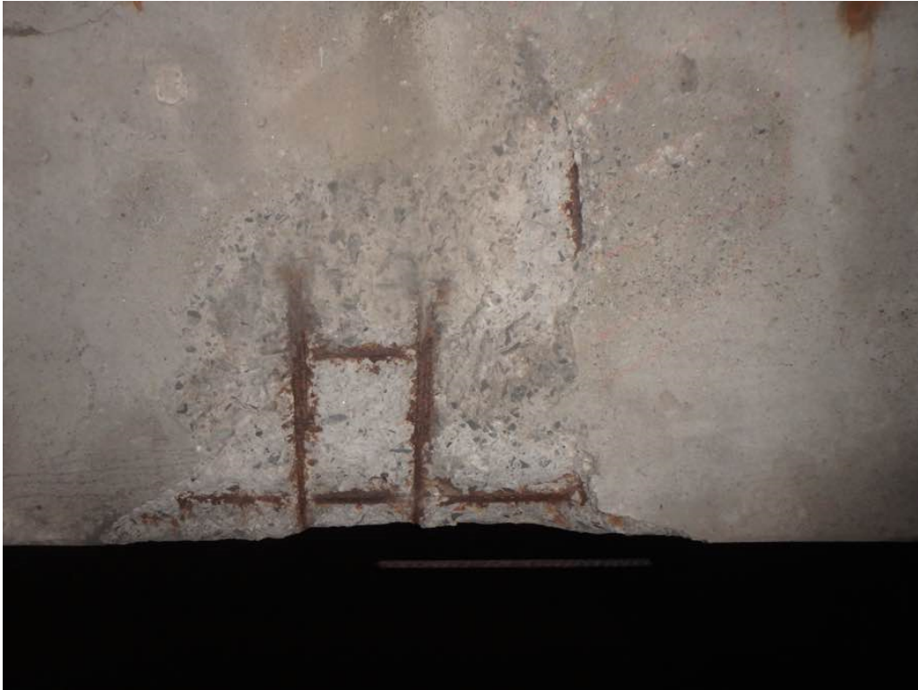
Photo 57: Moderate to heavy spalling with hollow concrete below and just to the east of Beam L at pier #1 cap north face
