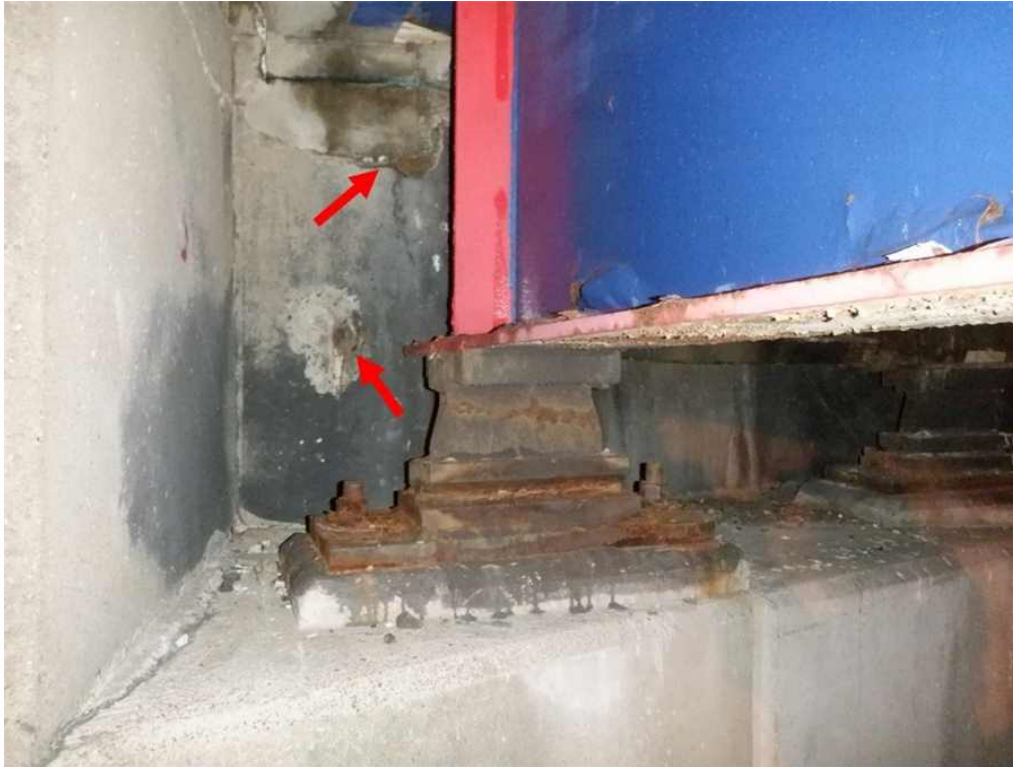
Photo 11: Beam 1G bearing, north abutment, looking north - heavy impacted rust. Note the minor spall with exposed rebar and crack with rust stains in the backwall.
