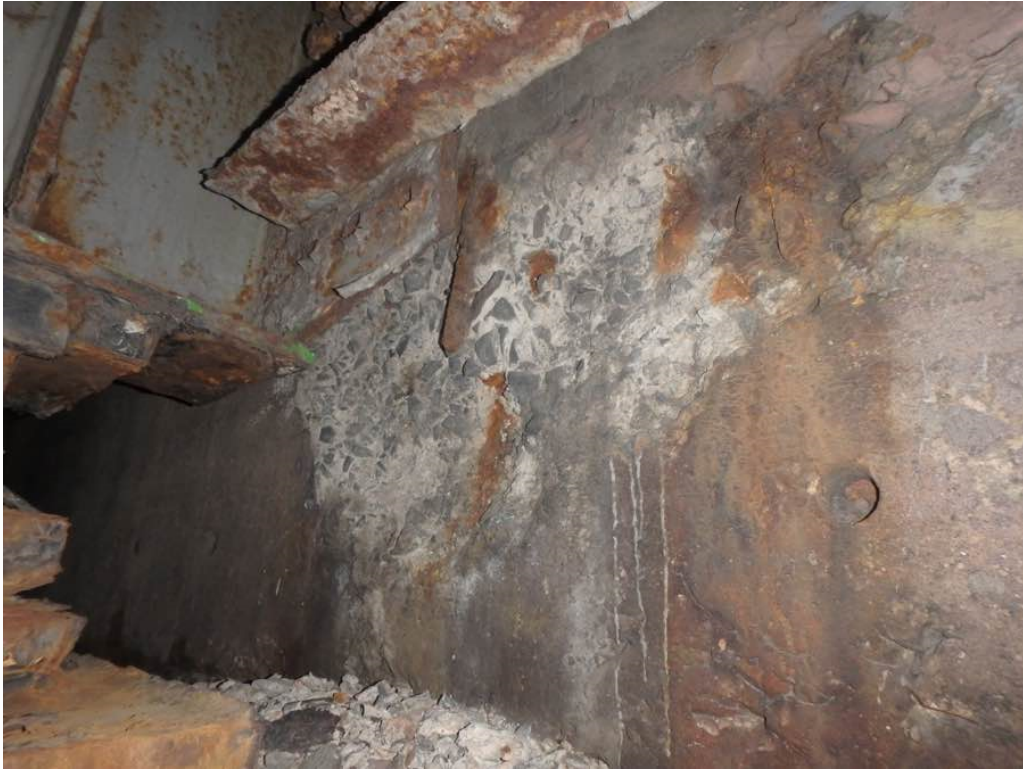
Photo 29: Moderate spalling at the top of the south backwall behind Beam P
