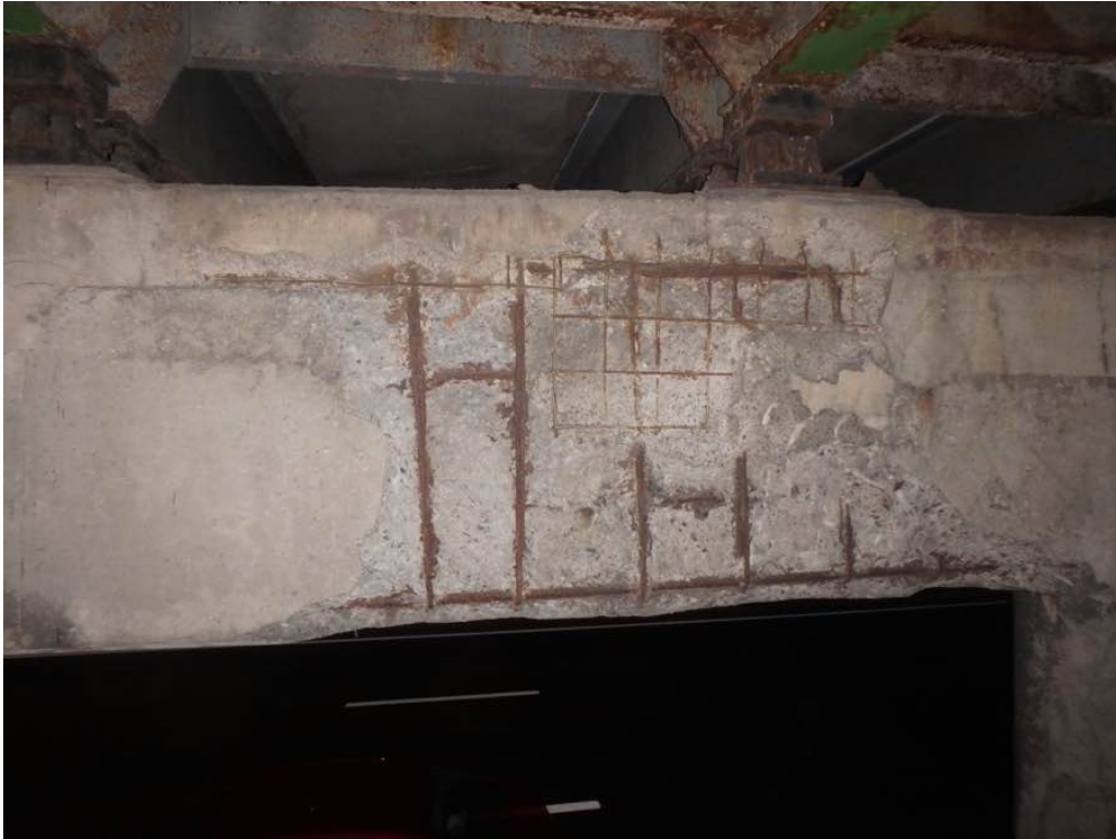
Photo 43: Heavy spalling with exposed rusted rebar at pier #1 cap south face full height between Beams C and D
