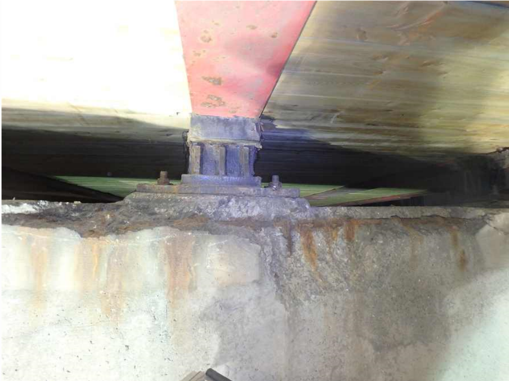
Photo 33: Pier 2 cap, north face below beam 2E, at the top, looking south - spall with exposed and debonded rebar that extends into the adjacent bays.
