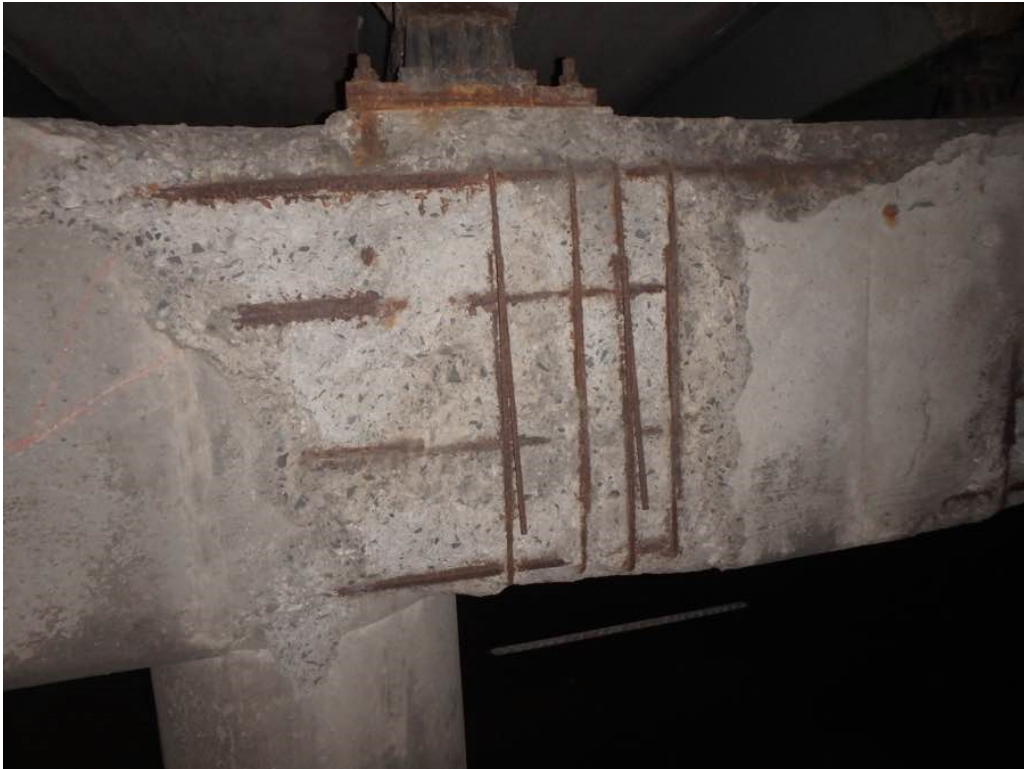
Photo 58: Heavy spalling with exposed rusted rebar at pier #1 cap north face between Beams L and N (mostly below beam M)
