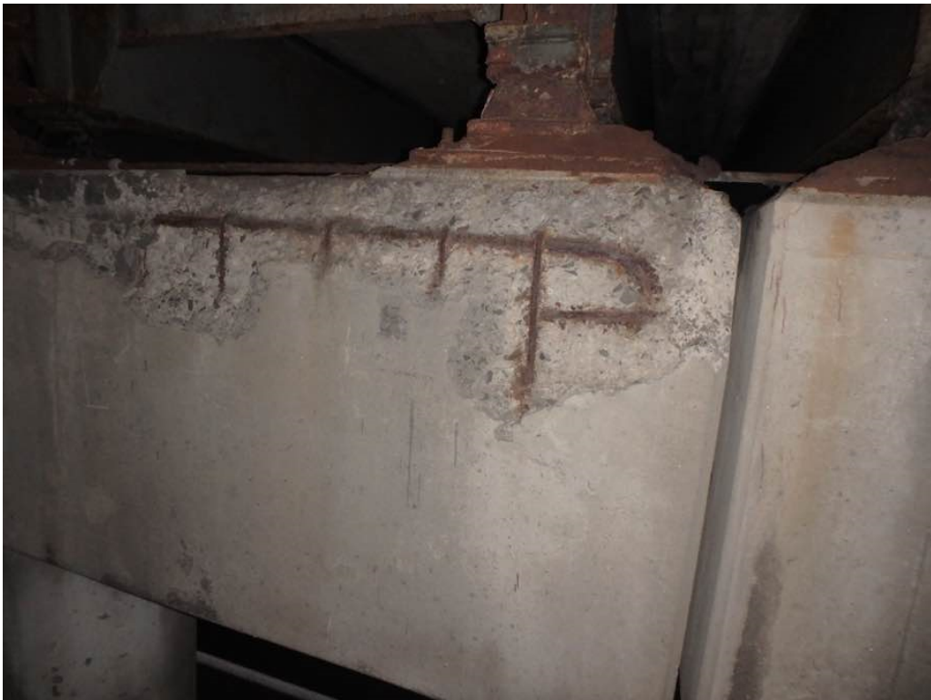
Photo 66: Moderate to heavy spalling with exposed rusted rebar at pier #2 cap north face between Beams J and K by Beam J
