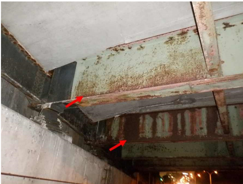
Photo 13: Span 1, north end, beams 1D and 1E bottom flanges and webs, looking east - paint loss, with moderate to heavy rust.
