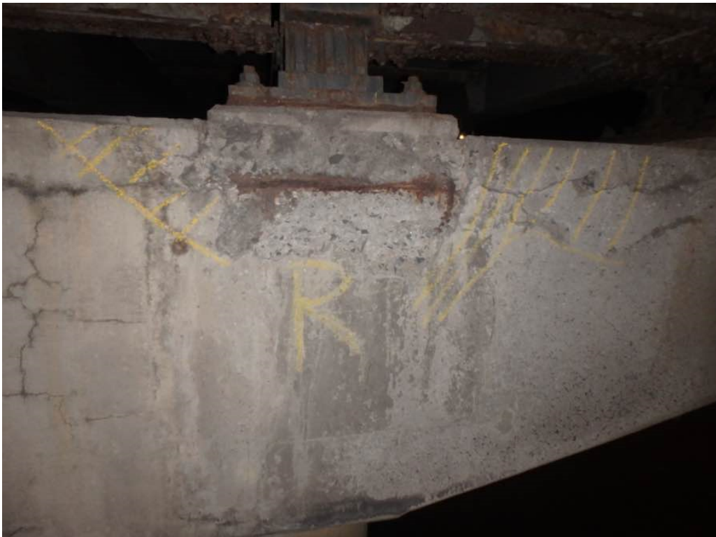
Photo 50: Moderate spalling with exposed rusted rebar at the top of pier #1 cap south face below Beam R and horizontal cracking and hollow concrete between Beams R and S
