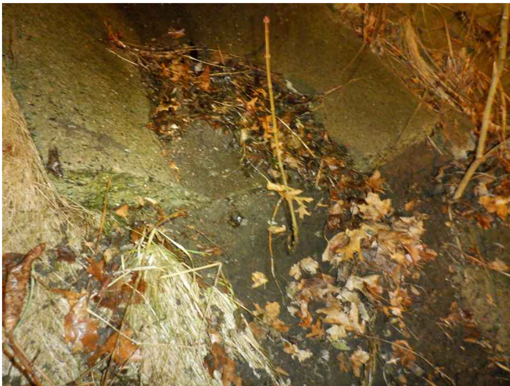
Photo 28: Concrete down trough, mid-height of the south embankment, east end looking south - through crack with settlement. Note the debris.
