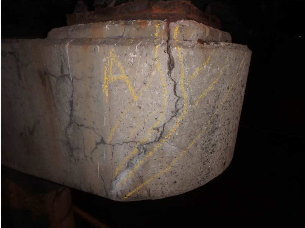
Photo 51: Moderate vertical crack at the west end of pier #1 cap on the north face
