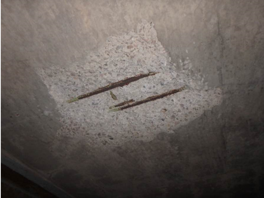
Photo 2: Moderate spalling in bay #11 in span #2 between the second interior diaphragm and pier #2
