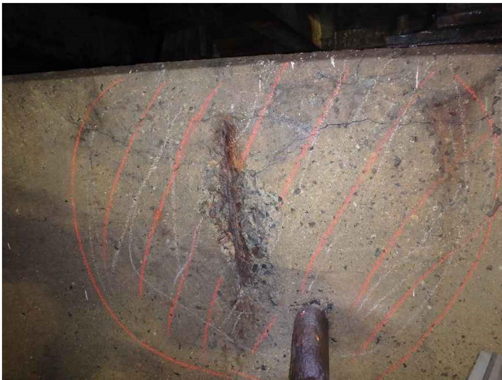
Photo 30: Pier 1 cap, south face between beams 2B and 2C, near beam 2B, at the top, looking north - spall with exposed rebar within a hollow area.
