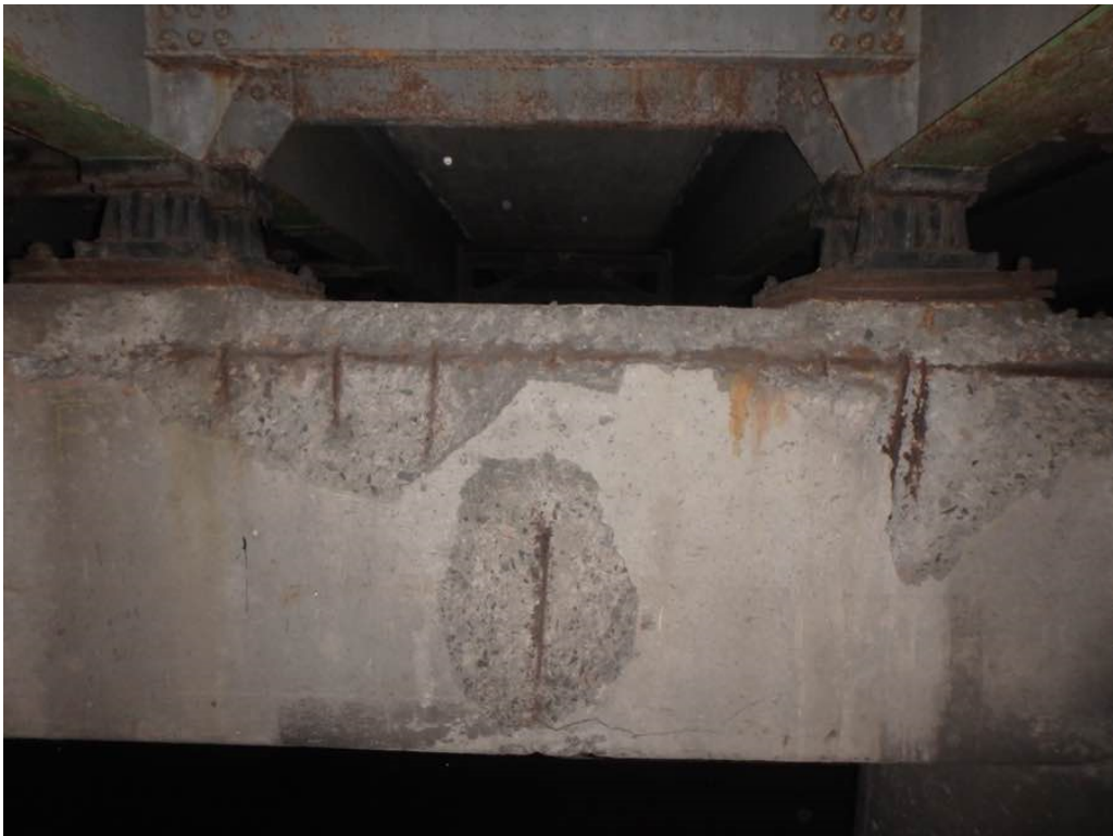
Photo 54: Heavy spalling with exposed rusted rebar at pier #1 cap north face between Beams E and F
