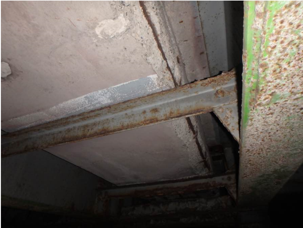
Photo 10: Spalling at the bottom east corner of the concrete encased utility duct in bay #2 in span #1 by pier #1
