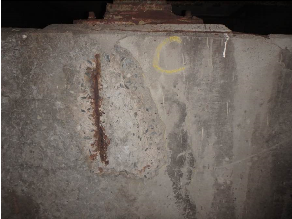
Photo 63: Moderate spall at pier #2 north face below Beam C
