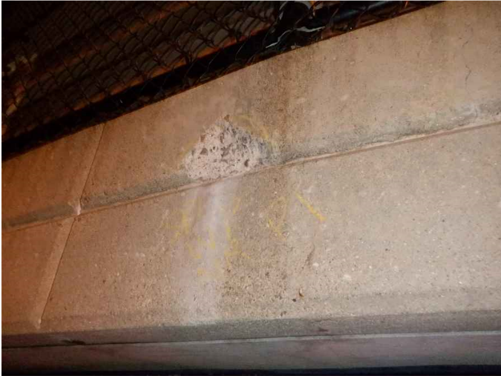
Photo 5: West sidewalk, in span 1, looking east - spall.
