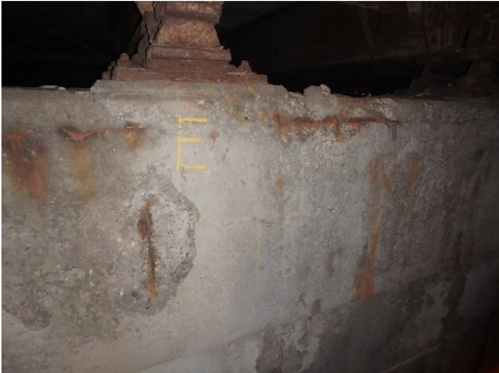
Photo 64: Moderate spalling with exposed rusted rebar at the top of pier #2 cap north face between Beams D and E by Beam E
