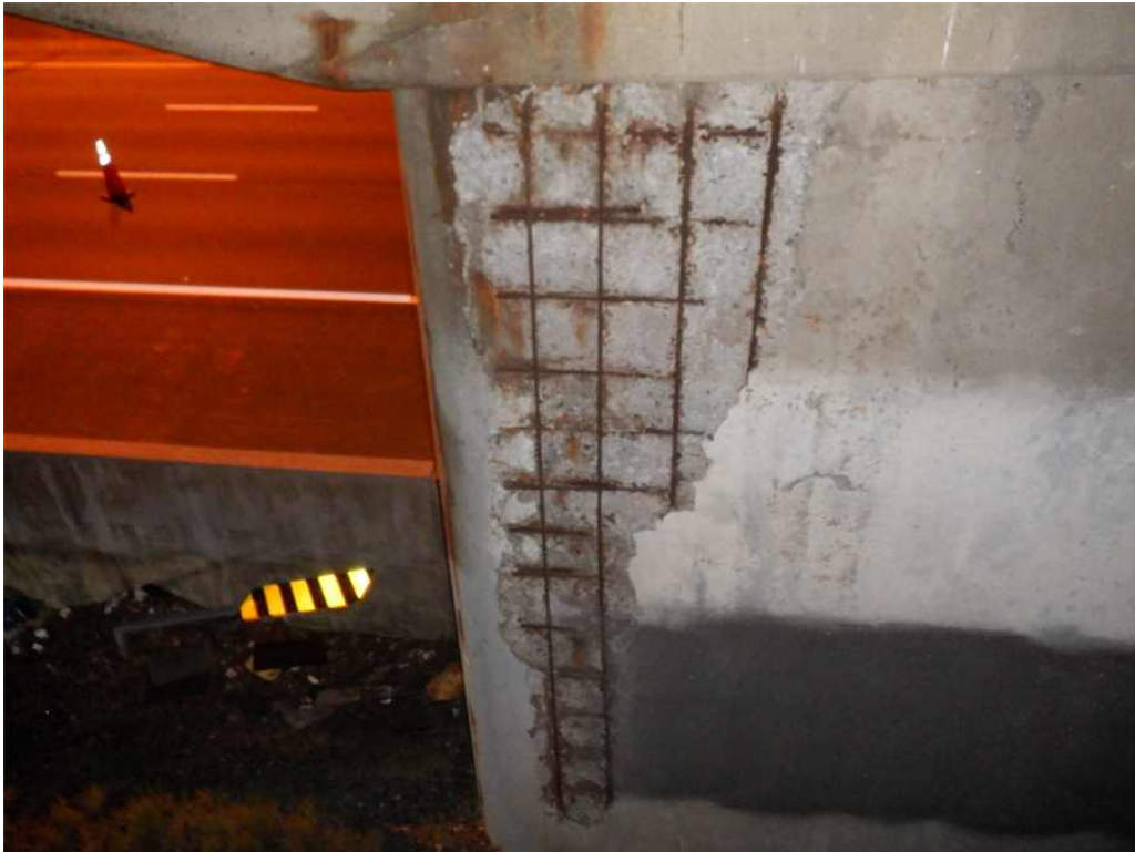
Photo 20: Pier 1, north face, east end, below beam 1B - up to full height spall with exposed, debonded, and deteriorated rebar.
