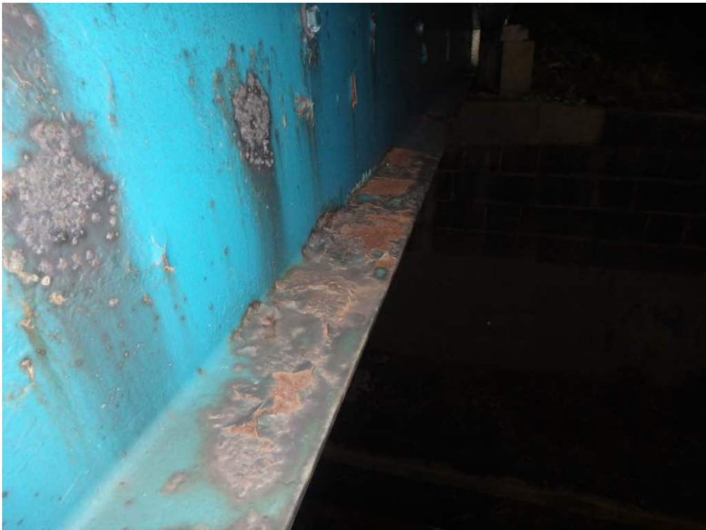
Photo 20: Peeling paint with lamination on the top face of the east leg of the bottom flange at Beam S in span #3
