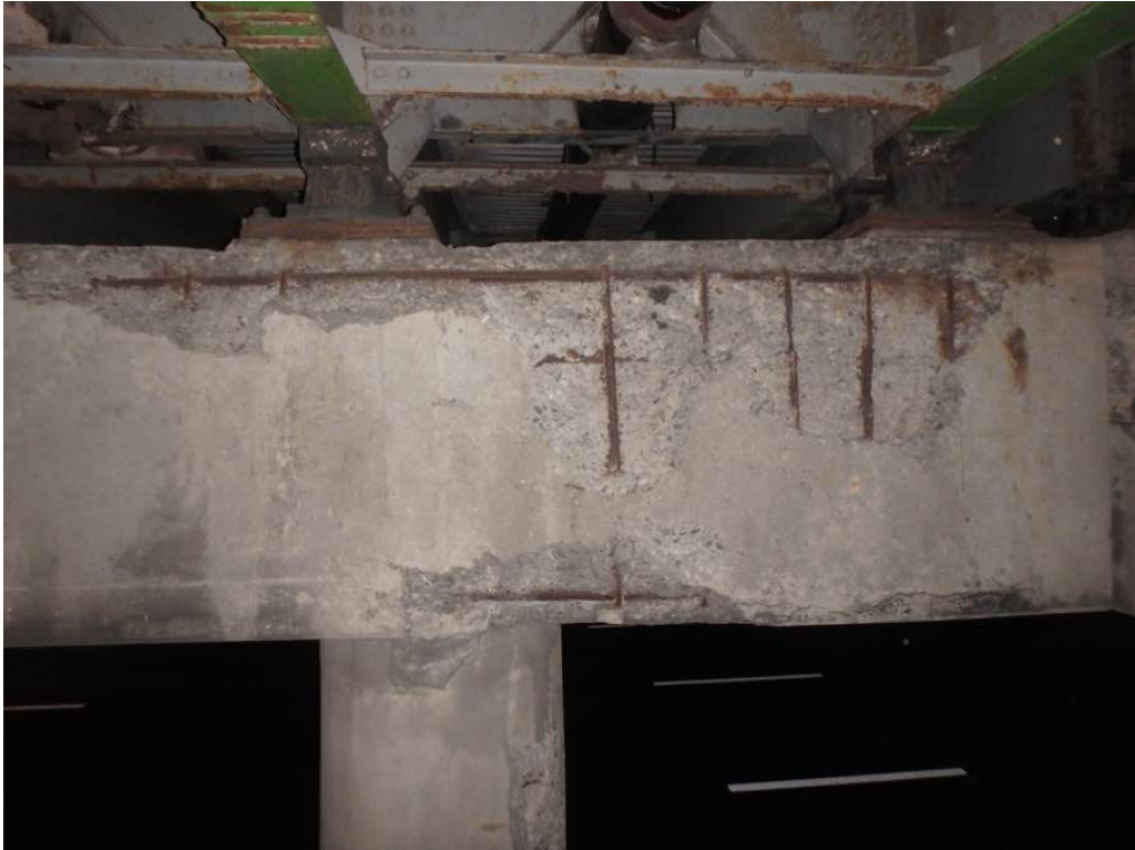
Photo 45: Heavy spalling with exposed rusted rebar at the top and bottom with horizontal cracking at the bottom of pier #1 cap south face between Beams G and H
