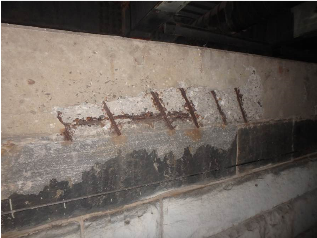
Photo 38: Heavy spalling with exposed rusted rebar and hollow concrete in the concrete cap at the north breastwall below Beam F
