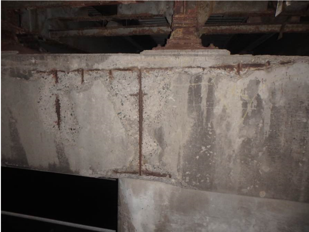
Photo 65: Heavy spalling with exposed rusted rebar at pier #2 cap north face below from just west of Beam G to west of Beam H
