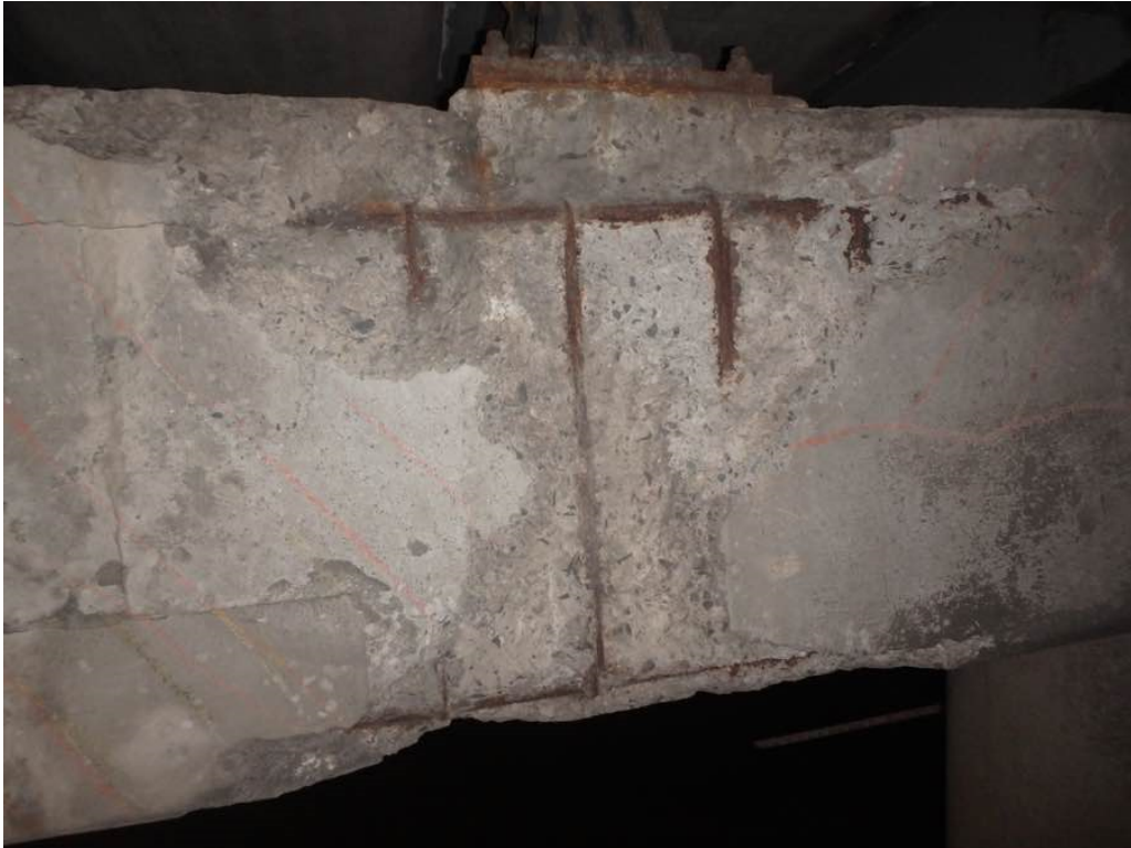
Photo 59: Heavy spalling at pier #1 cap north face below Beam N
