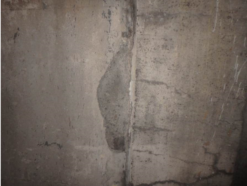
Photo 32: Minor spall and hollow concrete at the top of the south breastwall between Beams H and J
