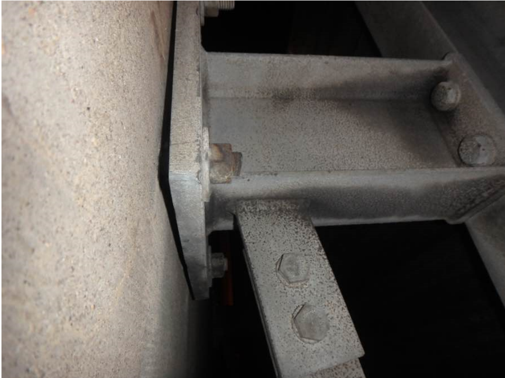
Photo 17: Gap (5/16") between the third horizontal support and east face of the deck in span #2
