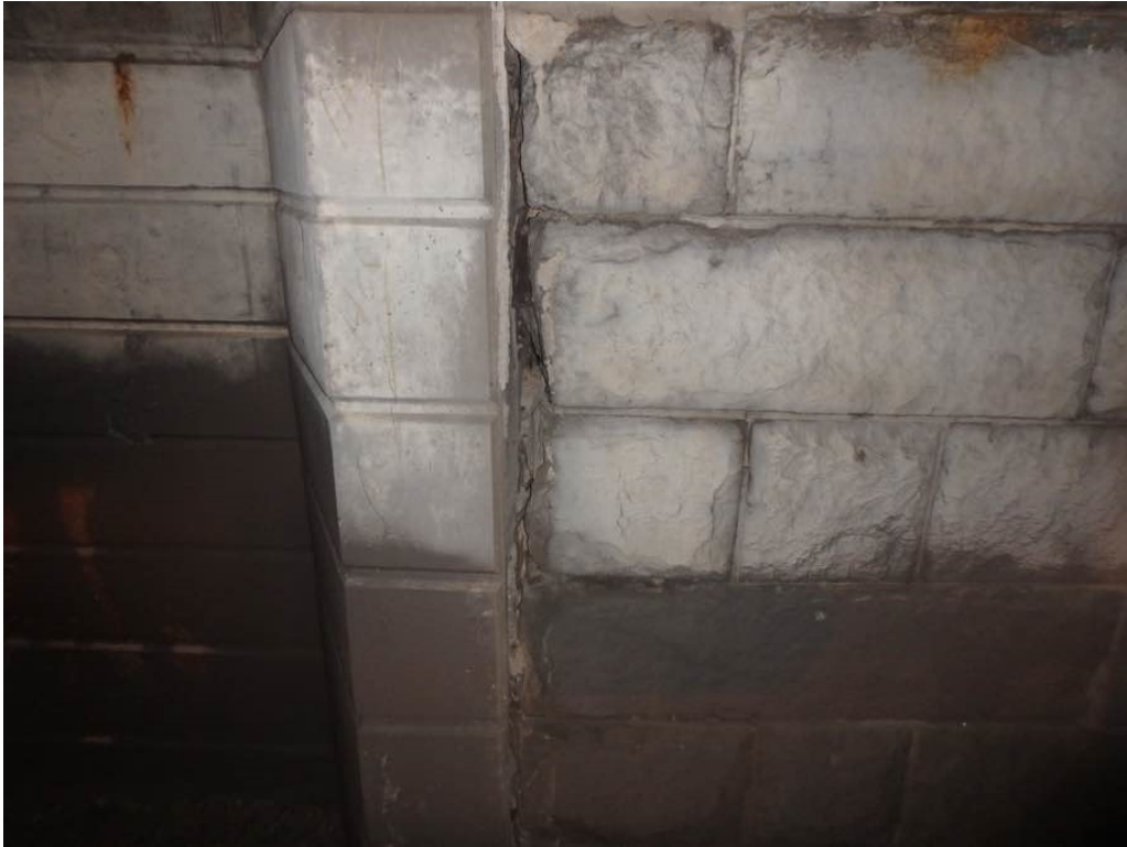
Photo 37: Void area between the concrete and masonry portions of the north breastwall between Beams D and E
