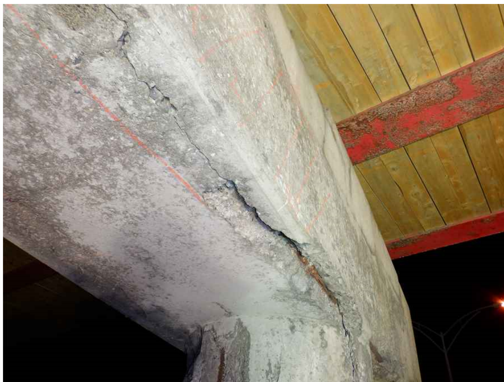
Photo 39: Pier 2 cap, between columns 1 and 2, looking up and southwest - along the north and south edges are hollow areas with longitudinal cracks and exposed rebar.
