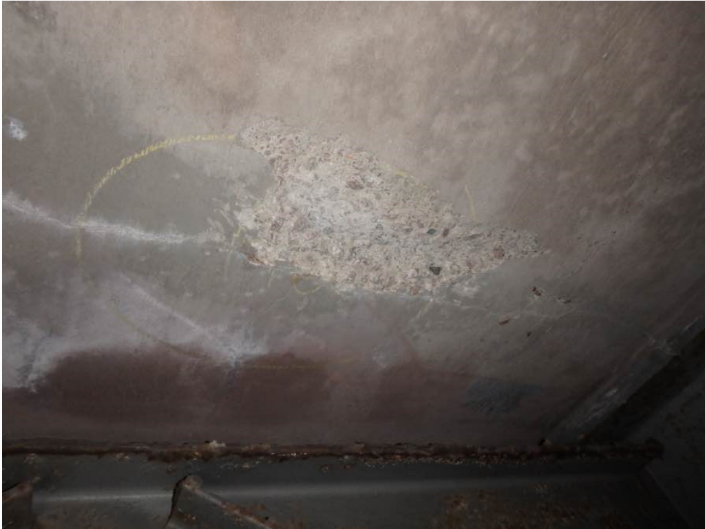
Photo 1: Light transverse crack with minor efflorescence, minor spalling, and hollow concrete in bay #11 in span #2 just north of the second interior diaphragm
