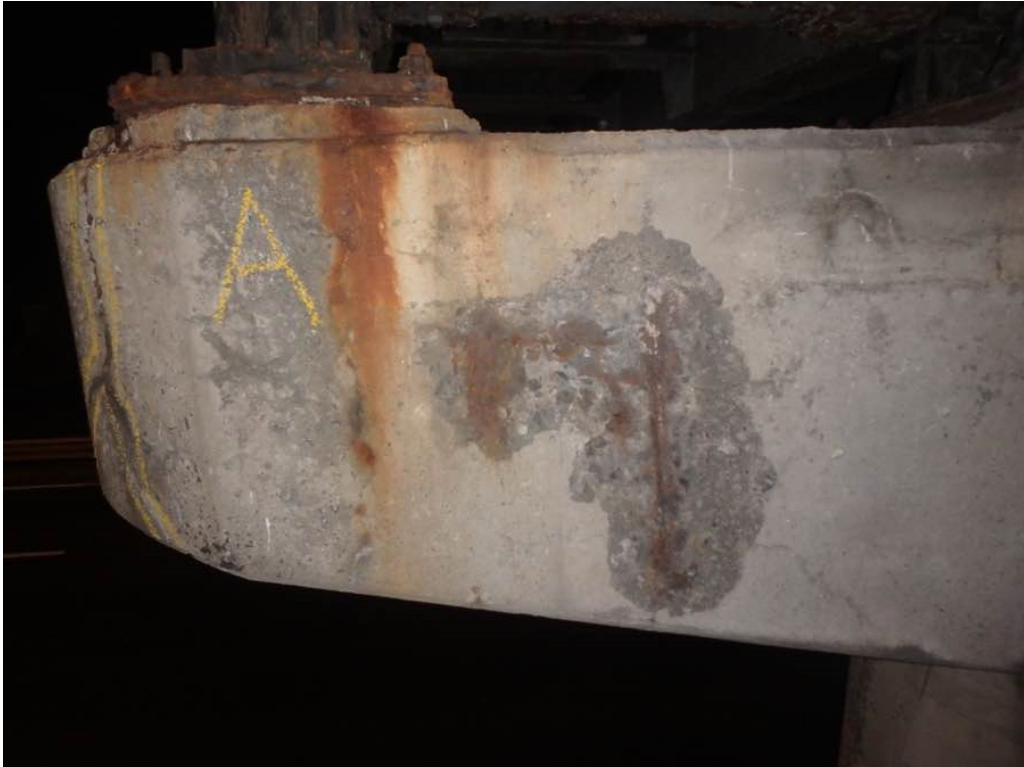
Photo 41: Moderate spalling with exposed rusted rebar and hollow concrete at pier #1 cap south face between Beams A and B
