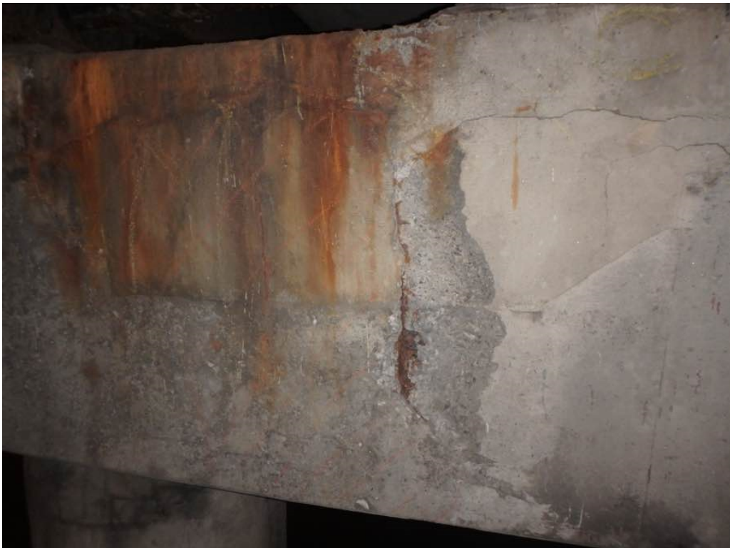
Photo 42: Hollow concrete with minor spalling at pier #1 cap south face between Beams B and C
