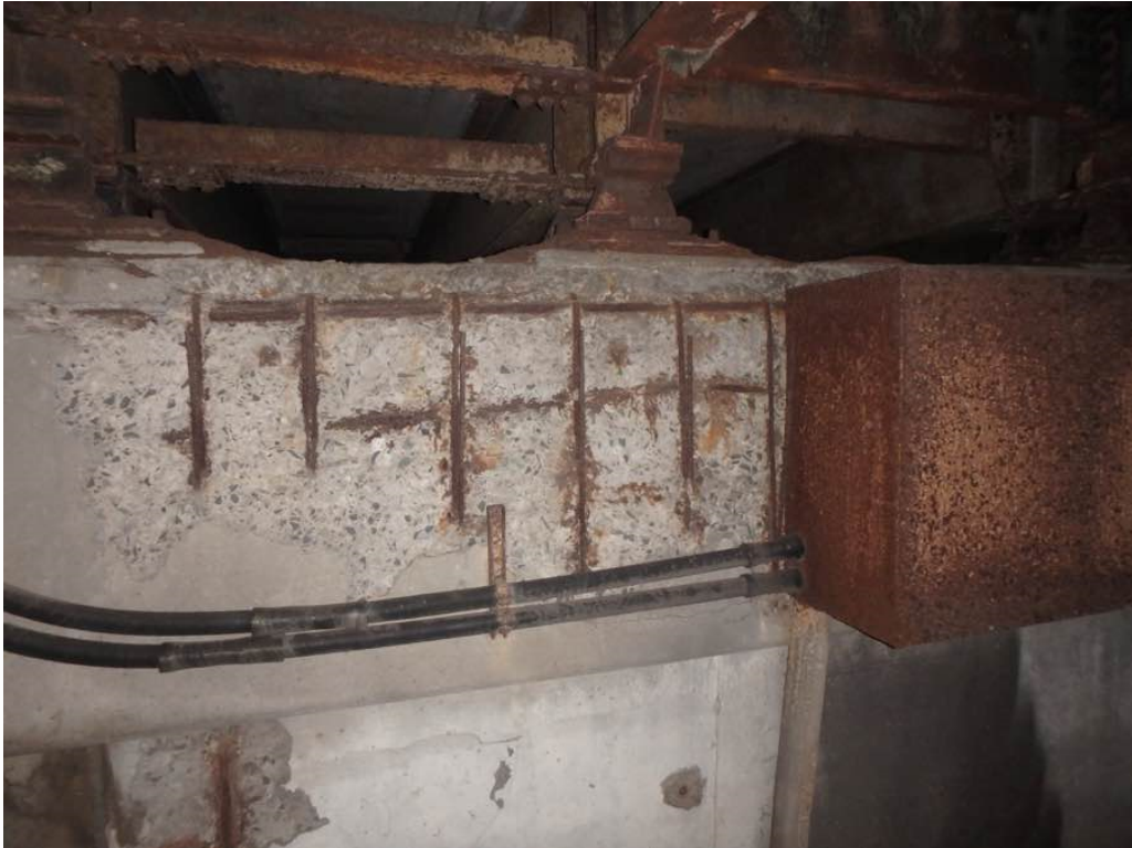
Photo 7: Heavy rusting of the junction box at pier #2 cap north face between Beams N and P
