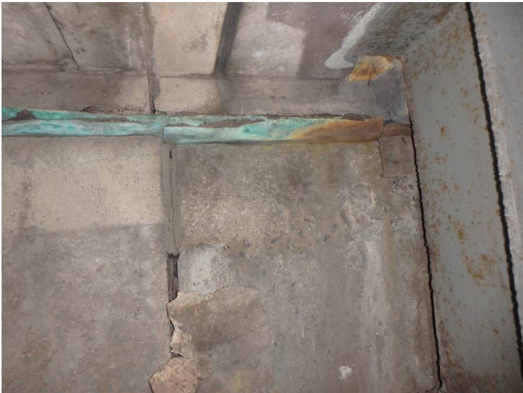
Photo 28: Moderate spalling at the top of the south backwall between Beams H and J by Beam H
