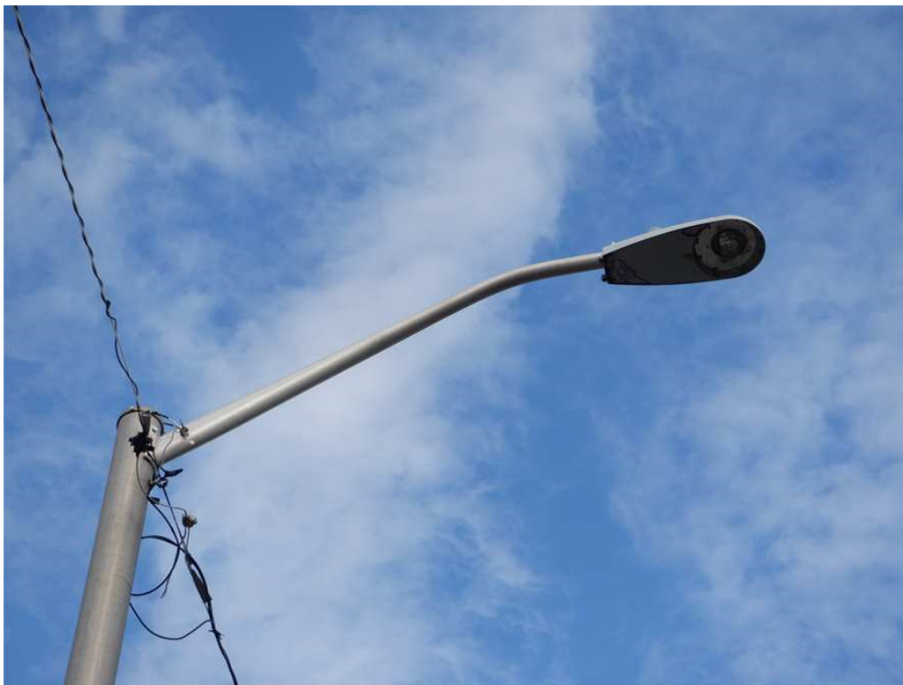
Photo 13: Lighting standard, span 2, west side near pier 1, looking north - missing luminaire.
