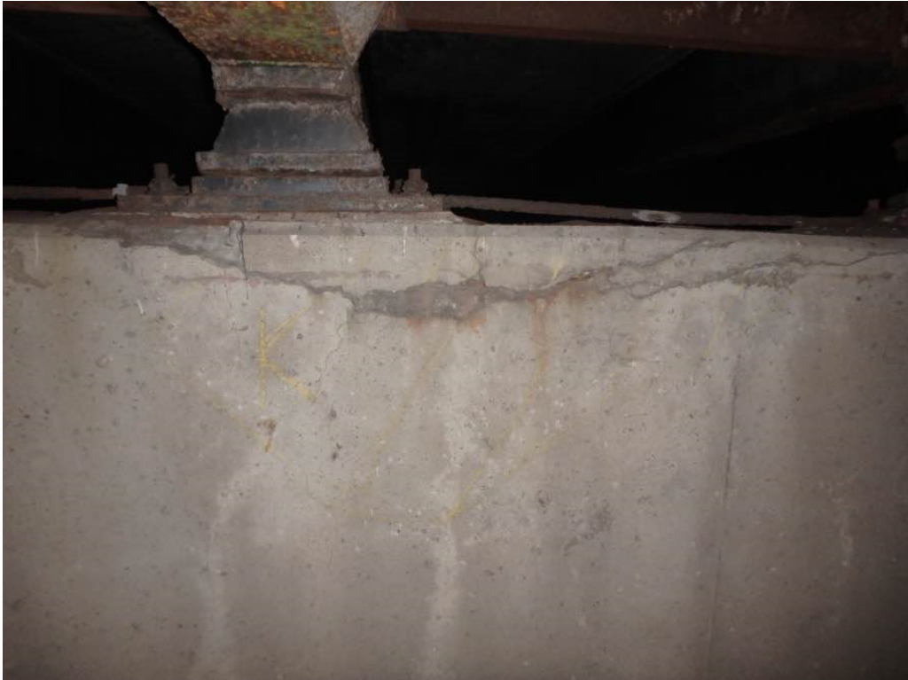
Photo 61: Horizontal cracking with minor spalling and hollow concrete at the top of pier #2 cap south face below and to the east of Beam K
