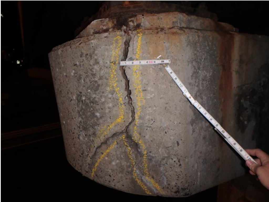
Photo 40: Heavy vertical crack (3/4" wide) at the west end of pier #1 cap at the south face
