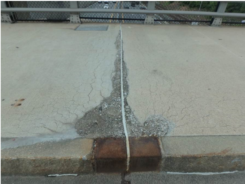
Photo 4: Minor to moderate scaling and hairline cracking in spans #1 and #2 at pier #1 at the west sidewalk
