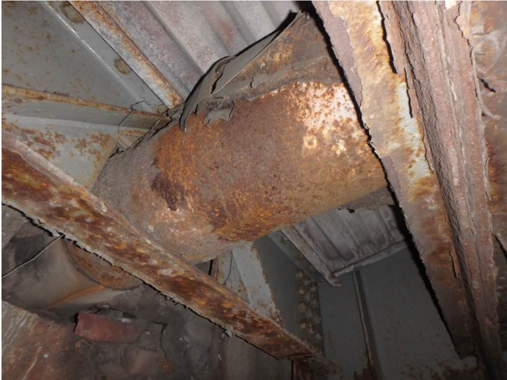
Photo 11: Heavy rusting of the utility pipe in bay #6 in span #1 at the south abutment
