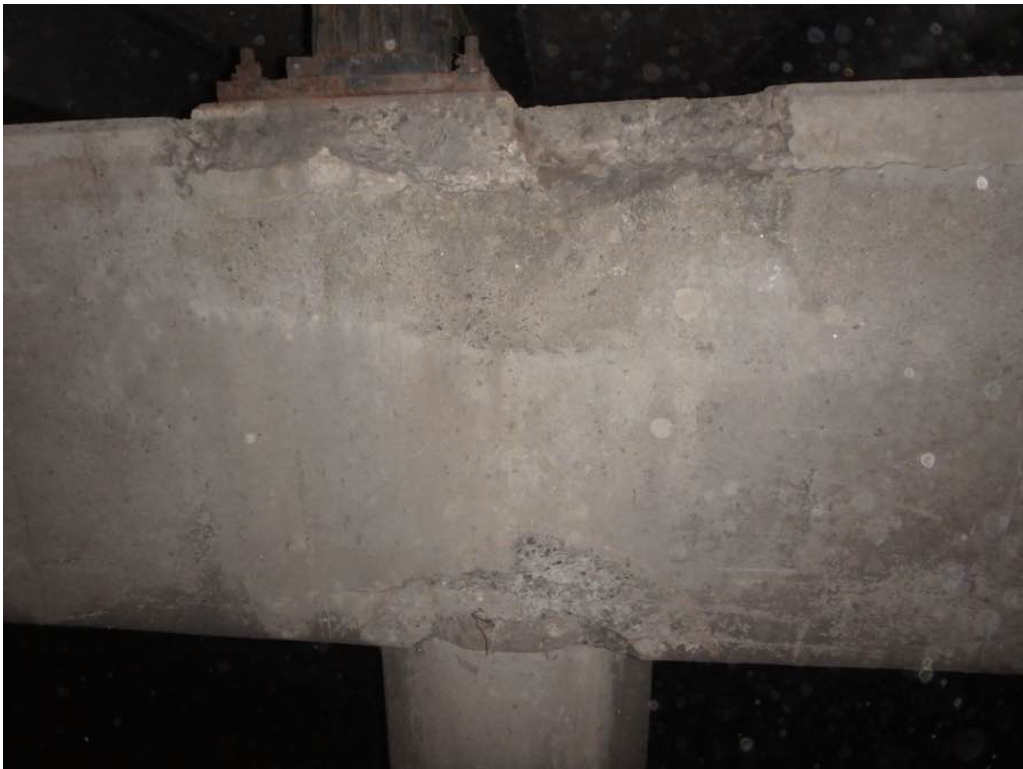
Photo 56: Moderate to heavy spalling with exposed rusted rebar at the top corner and minor spall at the bottom corner at pier #1 cap north face below Beam K
