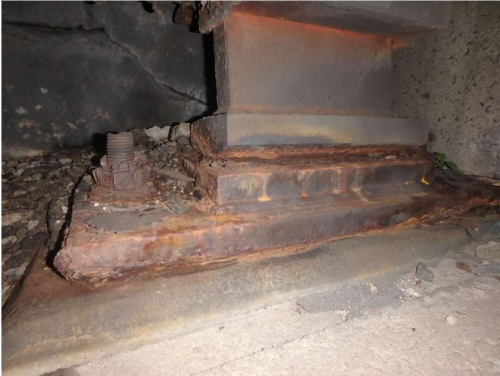
Photo 23: Impacted rust between the rocker and masonry plate at Beam S at the north abutment
