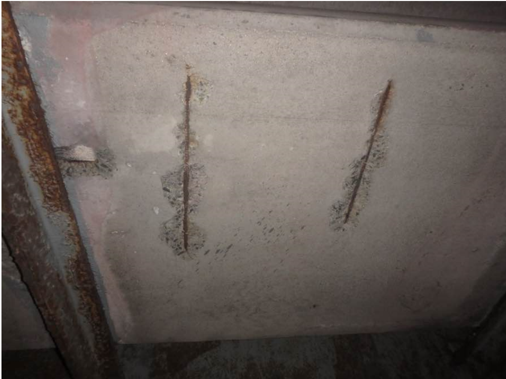
Photo 8: Minor spalls on the bottom face of the concrete encased utility duct in bay #2 in span #1 between the first and second utility supports from the south abutment
