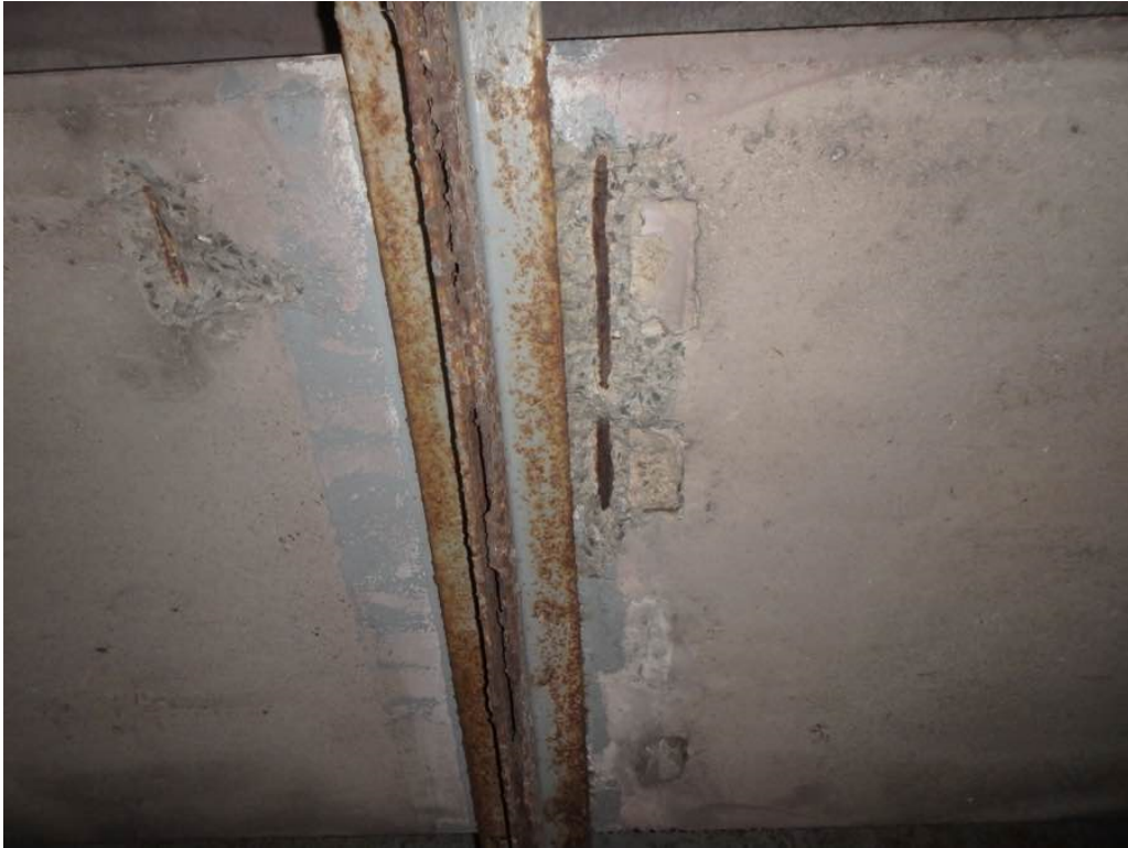
Photo 9: Minor spalls on the bottom face of the concrete encased utility duct in bay #2 in span #1 on the south and north sides of the third interior utility support from the south abutment
