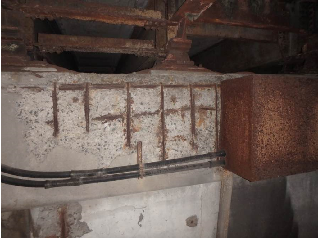
Photo 68: Heavy spalling with exposed rusted and debonded rebar at pier #2 cap north face between Beams P and R
