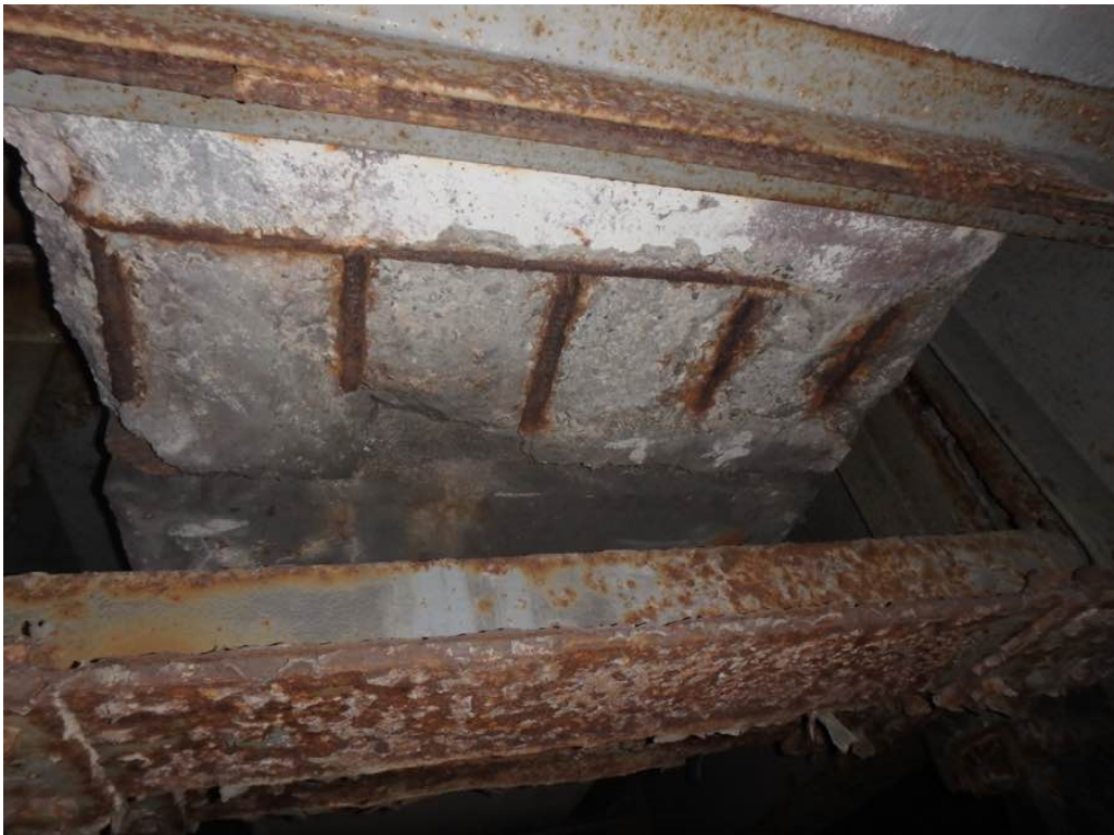
Photo 12: Moderate spalling on the bottom face of the concrete encased utility duct in bay #2 in span #2 at pier #1
