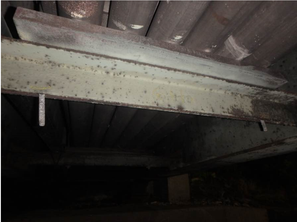
Photo 25: Missing nuts at the bottom of the sixth interior utility support in bay #15 in span #3
