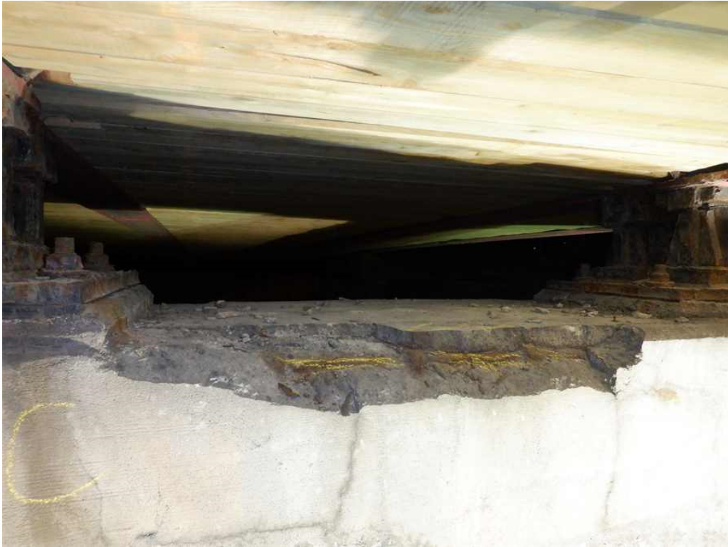
Photo 35: Pier 2 cap, south face between beams 3B and 3C, at the top, looking north - spall with exposed rebar. The remaining top concrete is hollow.
