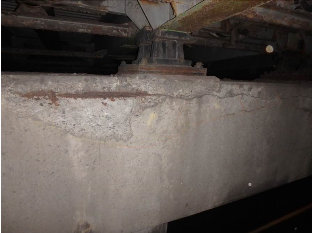
Photo 55: Horizontal cracking with hollow concrete/delamination between Beams F and G and spalling with horizontal cracking at the top corner of pier #1 cap north face just east of Beam G
