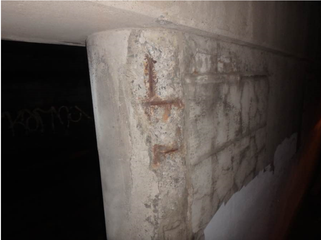
Photo 71: Moderate spalling on the south face of the pierwall at pier #2 east section below Beam K
