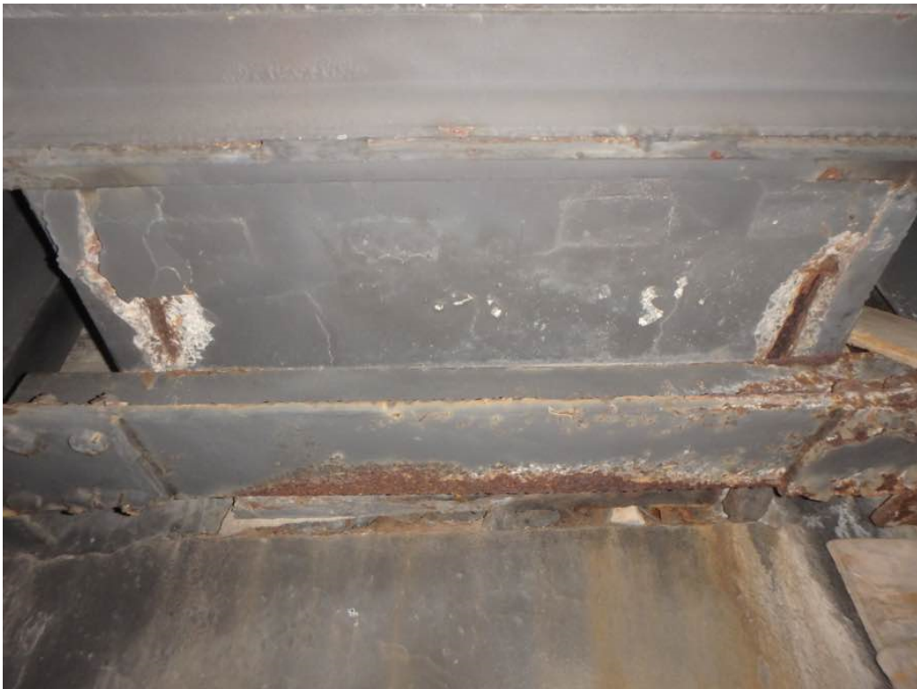
Photo 14: Minor spalling, cracking, and delamination on the bottom face of the concrete encased utility duct in span #3 at the north abutment
