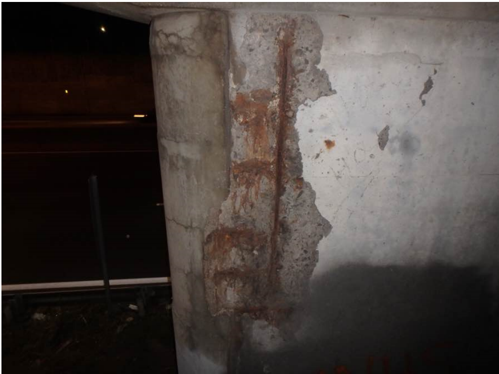
Photo 72: Moderate spalling with exposed rusted rebar at the top and hollow concrete at the bottom of the north face of the pierwall below Beam R
