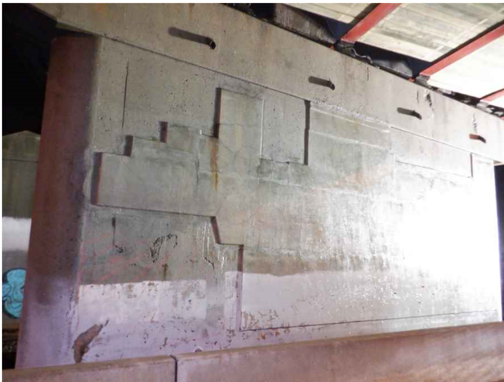
Photo 43: Pier 1, south face, looking north - typical cracked repair patches throughout.
