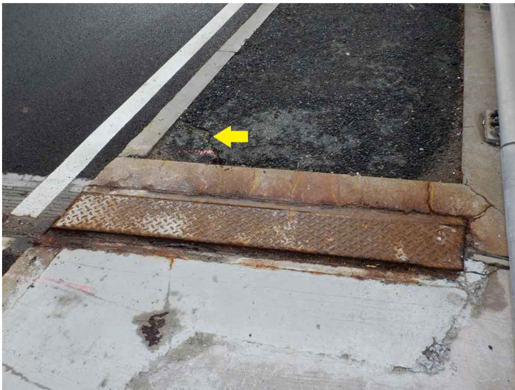
Photo 16: Southwest approach sidewalk, looking south - diagonal crack with minor settlement at the east edge of the sidewalk.
