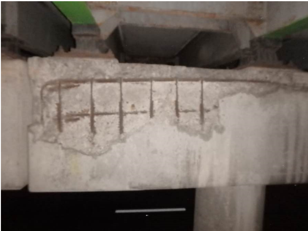
Photo 46: Heavy spalling with exposed rusted rebar and hollow concrete of pier #1 cap south face between Beams J and K
