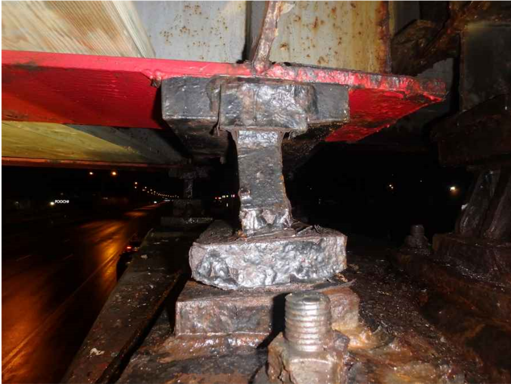
Photo 23: Beam 2B, span 2 at pier 1, looking west - the bearing is slightly contracted to the south.
