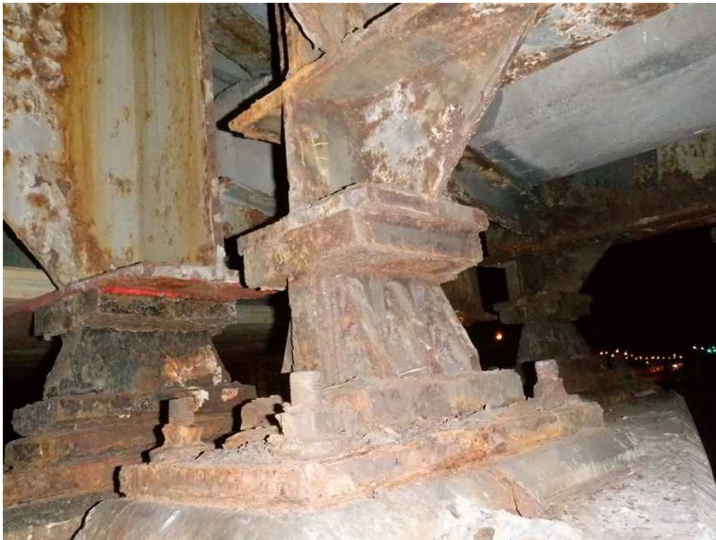
Photo 12: Beam 1F bearing, span 1, at pier 1, looking southwest - heavy rust and missing keeper plate.
