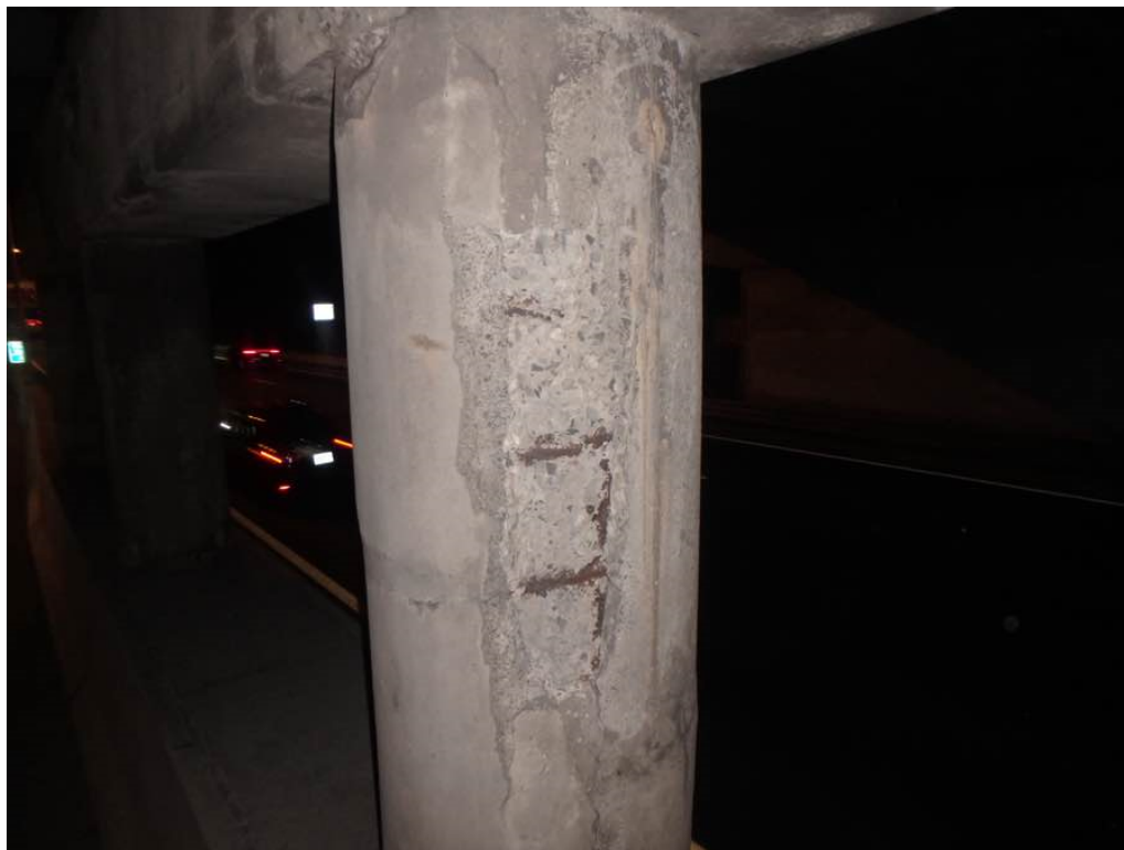
Photo 69: Light to moderate cracking and hollow concrete on the east face of column #3 at pier #1
