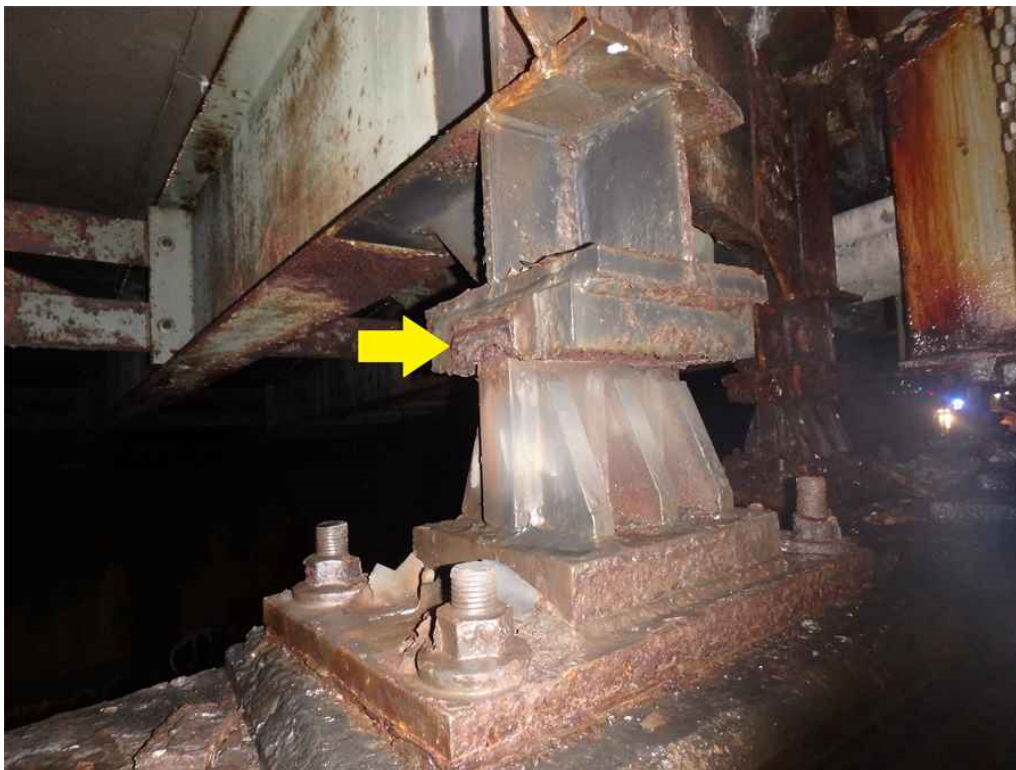
Photo 21: Beam 1C, span 1 at pier 1, looking northeast - the west keeper plate is missing.
