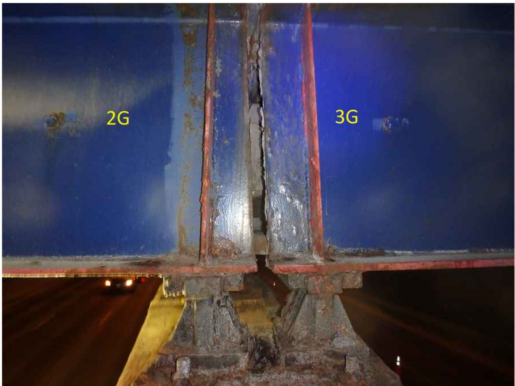
Photo 17: Beam 2G and 3G ends at pier 2, looking east - light rust with areas of pitting.
