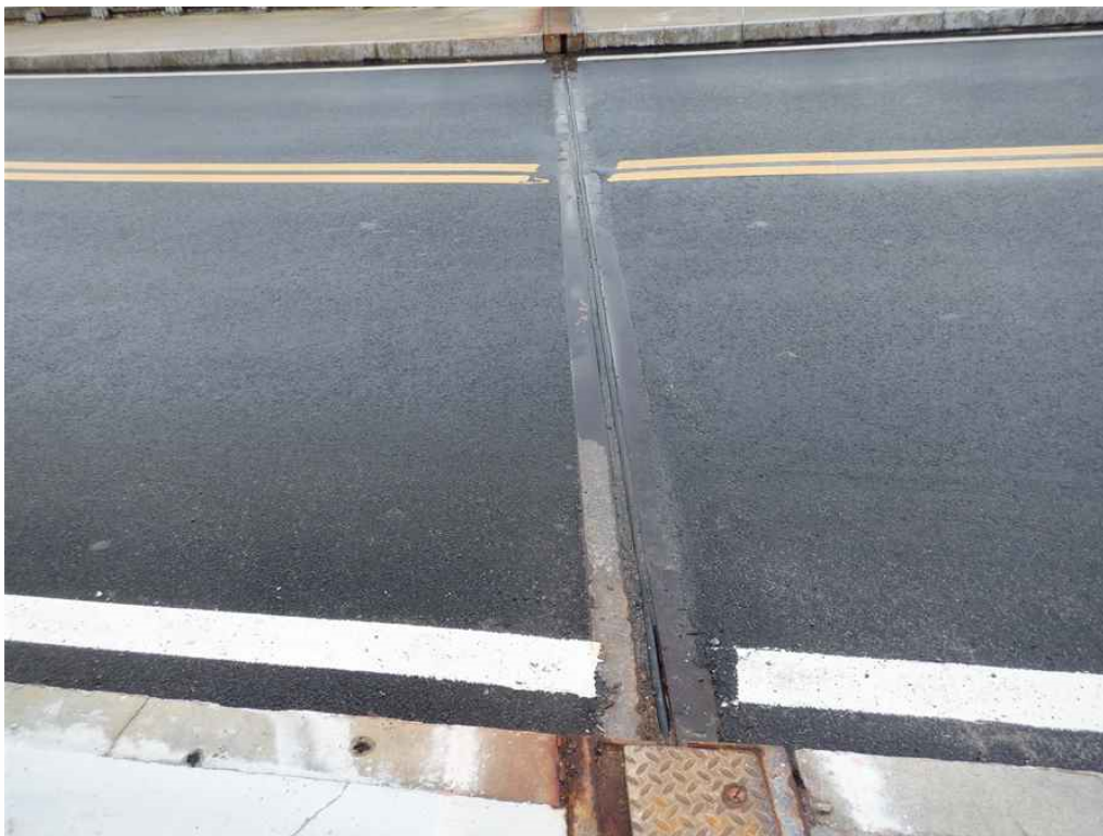
Photo 15: Pier 1 deck joint, looking east - previously noted deficiencies have been repaired.
