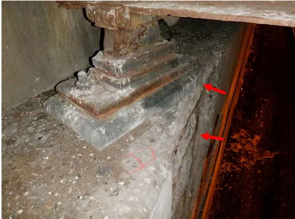
Photo 10: Beam 1D bearing, north abutment - unsupported at the east edge. Note the bridge seat and breastwall have spalls with exposed rebar.
