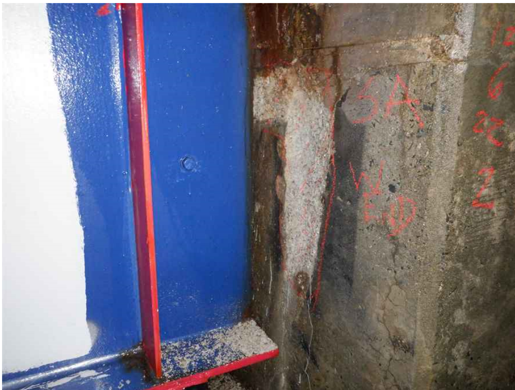
Photo 26: South abutment backwall behind beam 3G, near the top, looking southeast - area of scaling.
