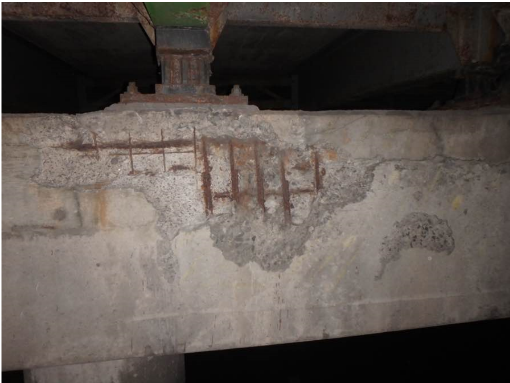
Photo 44: Heavy spalling with exposed rusted rebar and hollow concrete at pier #1 cap south face at the top below Beam E and between Beams E and F
