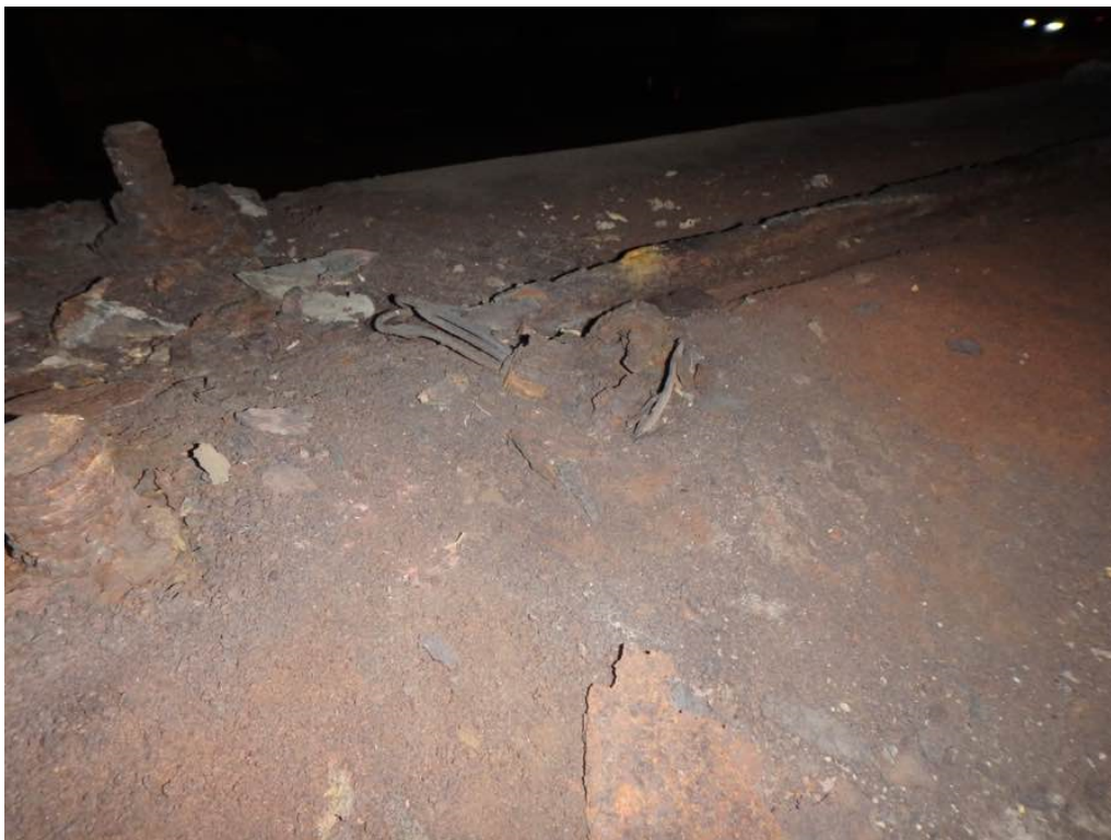
Photo 6: Area of 100% section loss with wires exposed on the top face of pier #2 cap top face just west of Beam P
