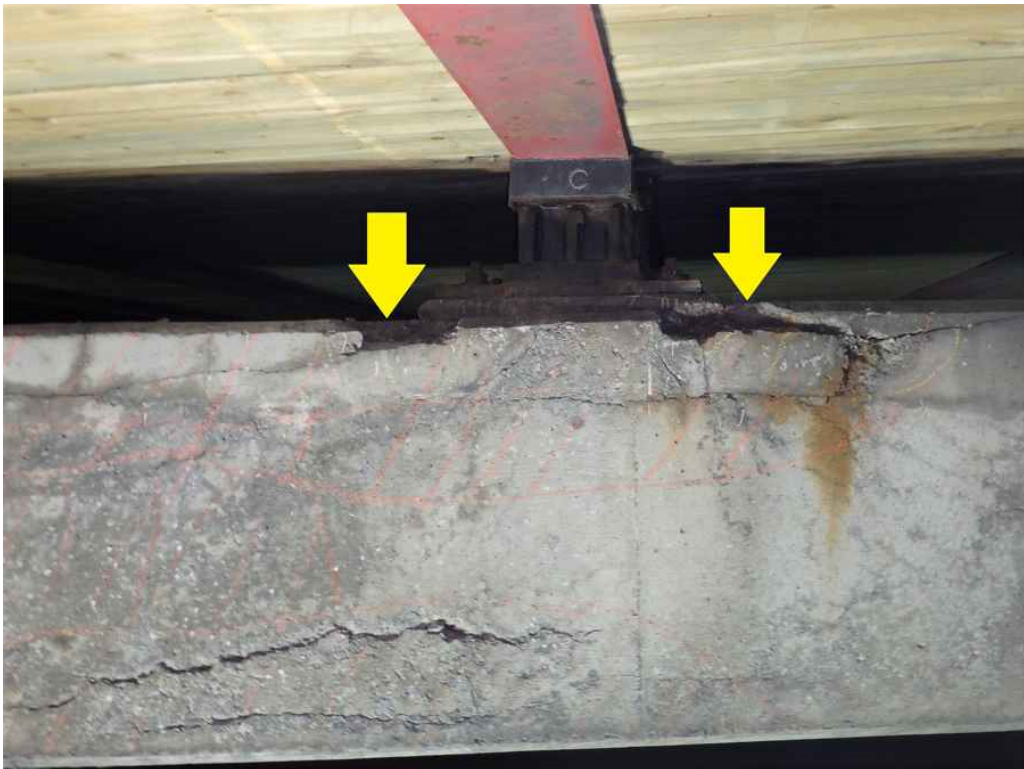
Photo 32: Pier 2 cap, north face below beam 2C, at the top and bottom, looking south - horizontal cracks with rust stains, top spalls in the previous repairs, and hollow areas.
