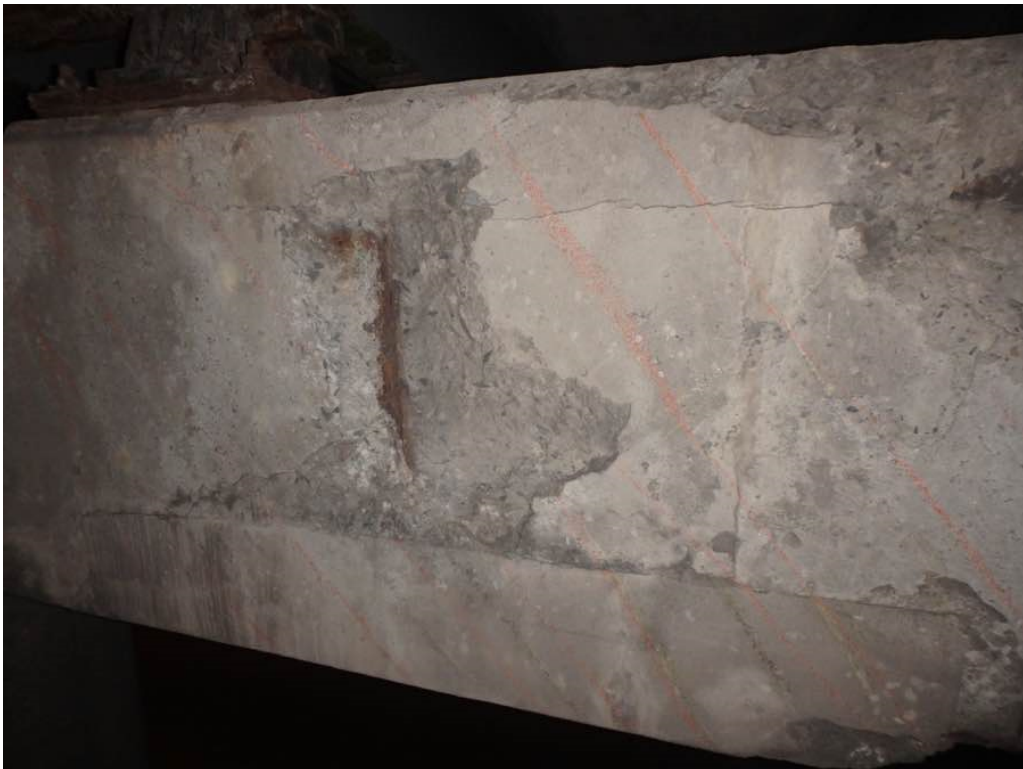
Photo 60: Moderate spalling with hollow concrete at pier #1 cap between Beams N and P
