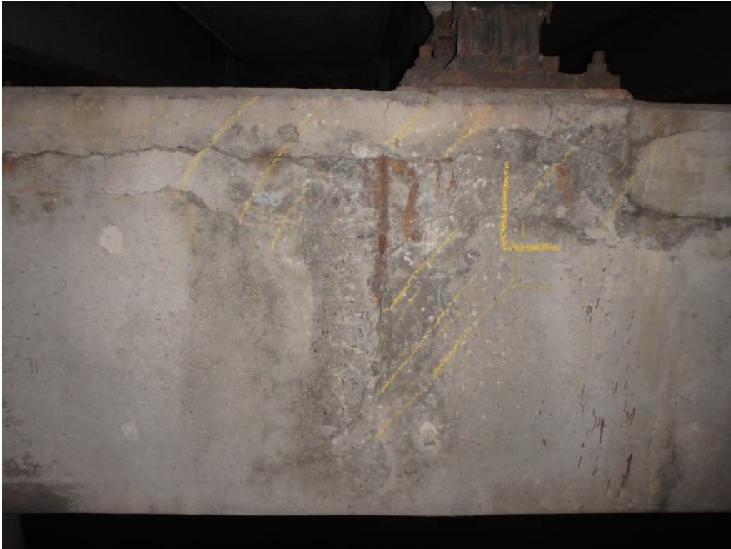
Photo 47: Moderate spall with exposed rusted rebar and hollow concrete at pier #1 cap south face just west of Beam L
