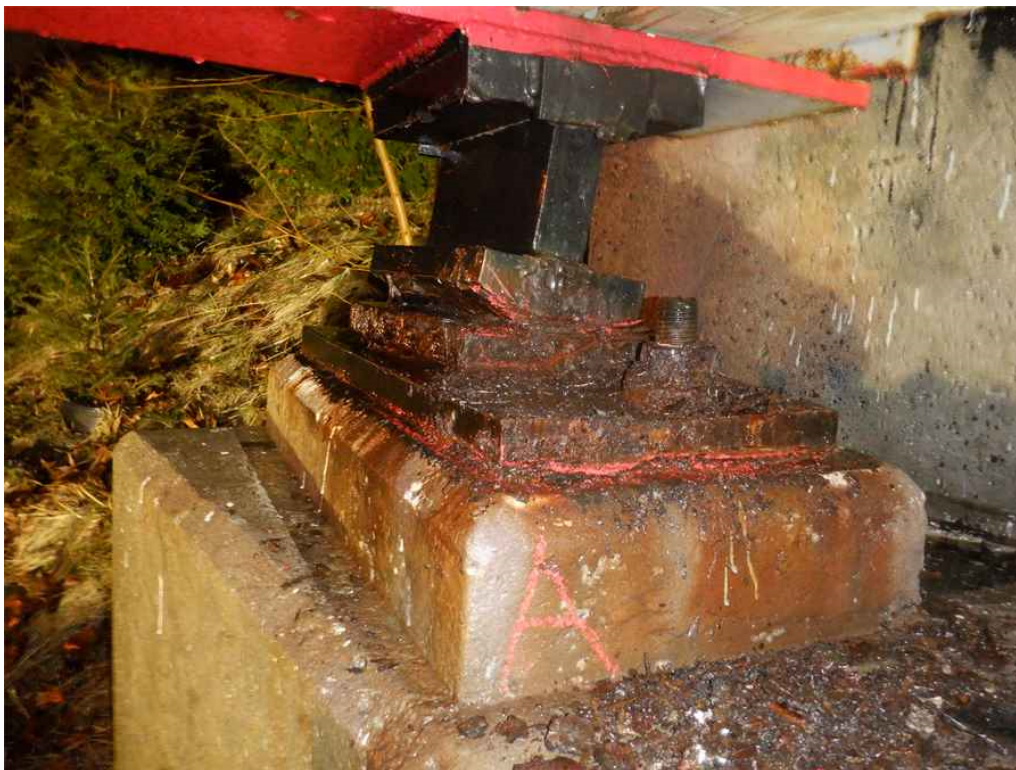
Photo 25: Beam 3A bearing, span 3 at the south abutment, looking southeast - impacted rust between the rocker and masonry plate.
