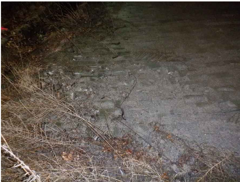
Photo 27: South embankment, east end, near mid-height, looking south - area of heavily deteriorated paving stones.
