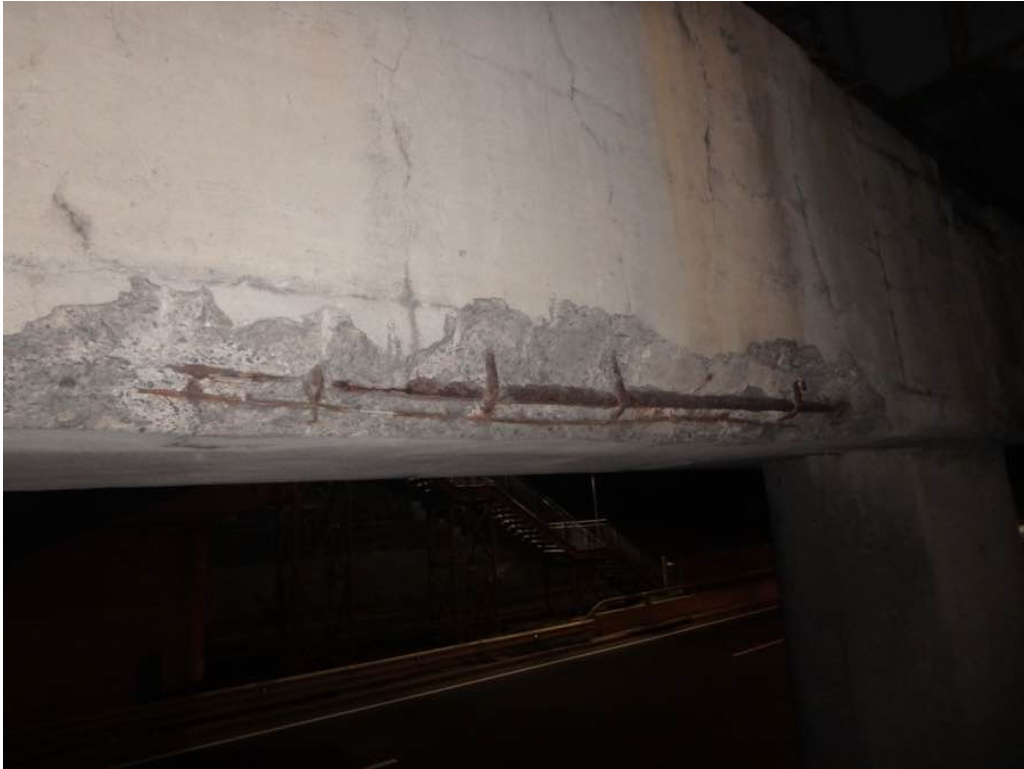
Photo 49: Moderate to heavy spalling with exposed rusted rebar at the bottom corner of pier #1 cap south face between Beams N and P
