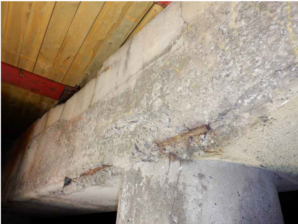
Photo 34: Pier 2 cap, south face between beams 3A and 3C, looking northwest - hollow area with several spalls with exposed rebar.
