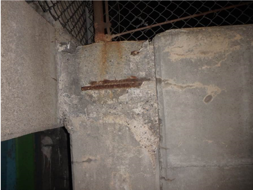
Photo 27: Moderate spalling at the top of the south backwall outside Beam A
