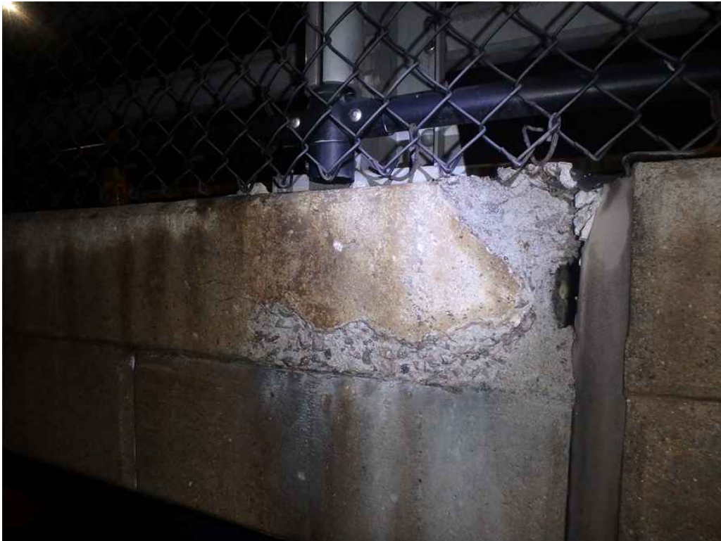
Photo 6: West sidewalk, span 1, at the pier 1 deck joint, looking east - spall/ heavy scale on the exterior face.
