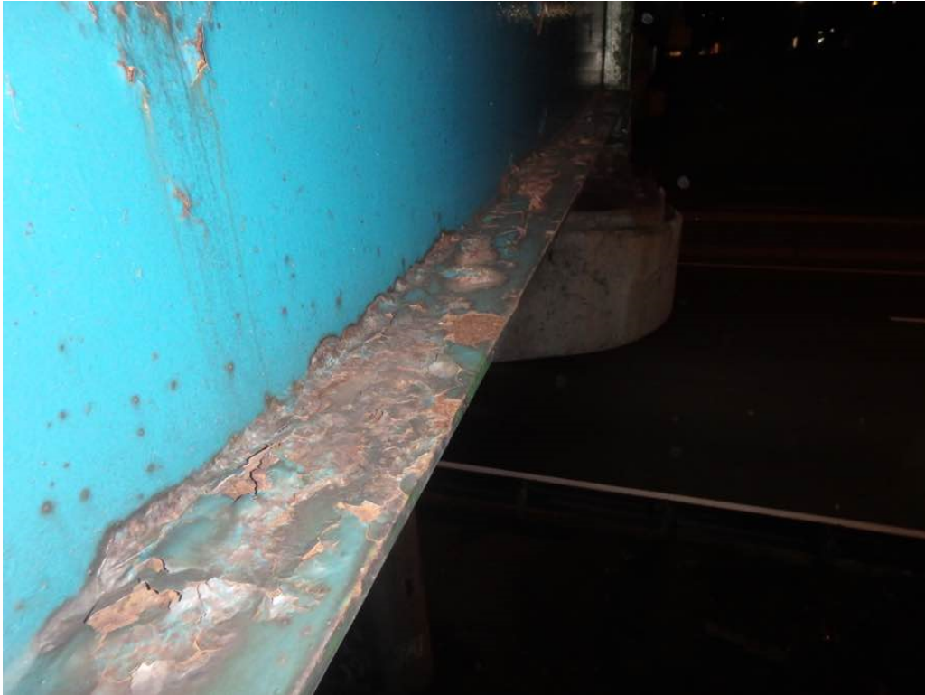
Photo 19: Peeling paint with lamination on the top face of the west leg of the bottom flange at Beam A in span #3
