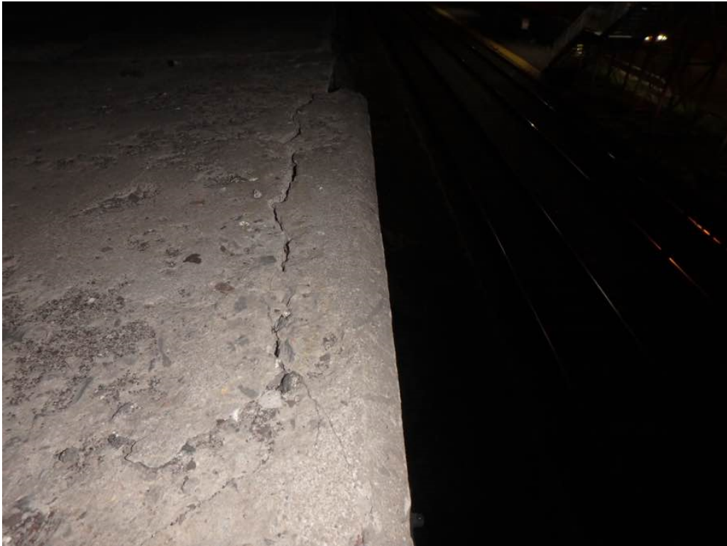
Photo 26: Heavy cracking and delamination at the edge of the north bridge seat between Beams L and M
