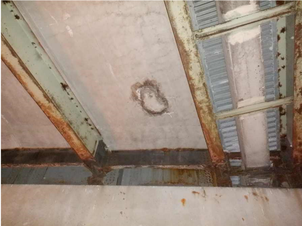
Photo 3: Underside of deck, span 1, at pier 1, in bay 5, looking south - moderate efflorescence at a repaired patch.
