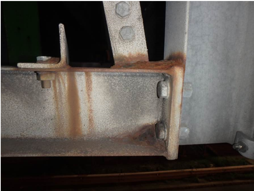
Photo 18: Typical rusting of the welded connections at the bottom horizontal support for the overhead sign in span #2
