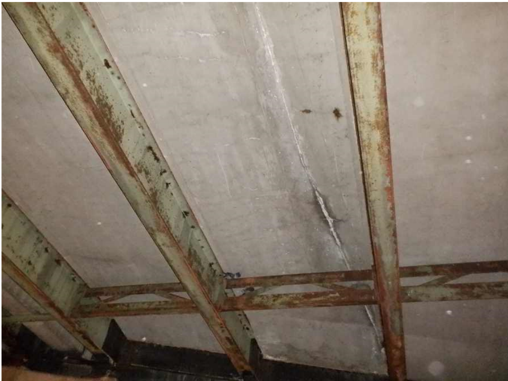
Photo 2: Underside of deck, span 1, in bay 4, just south of first interior diaphragm, looking north - heavy efflorescence at longitudinal cold joint.
