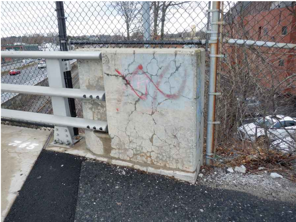
Photo 12: Southeast endpost, looking east - areas of map cracks throughout.
