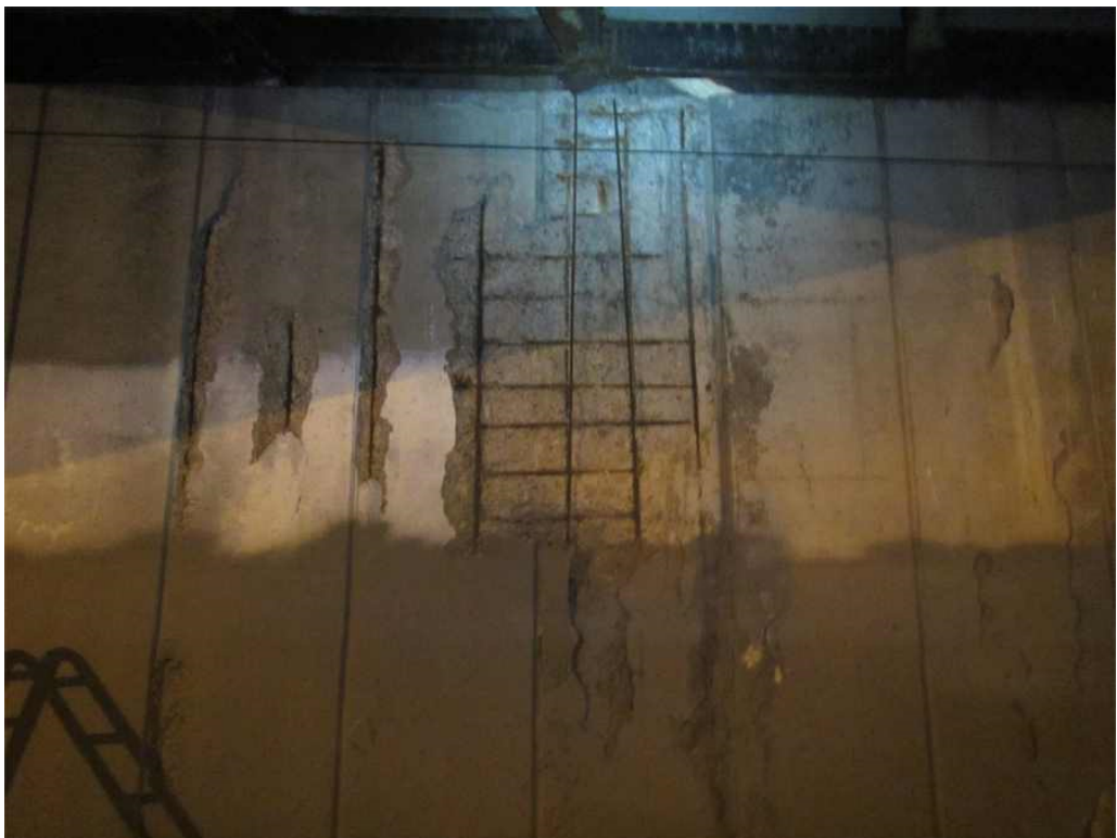
Photo 17: North abutment breastwall, between beam 1C and 1E - large spall with debonded rebars and adjacent delamination.
