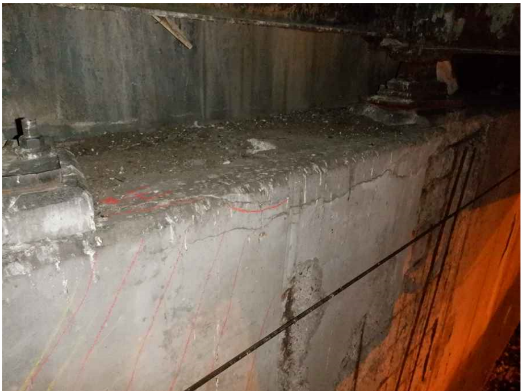
Photo 15: North abutment bridge seat, between beam 1D and 1E, looking northeast - hollow sounding concrete and cracks with efflorescence.
