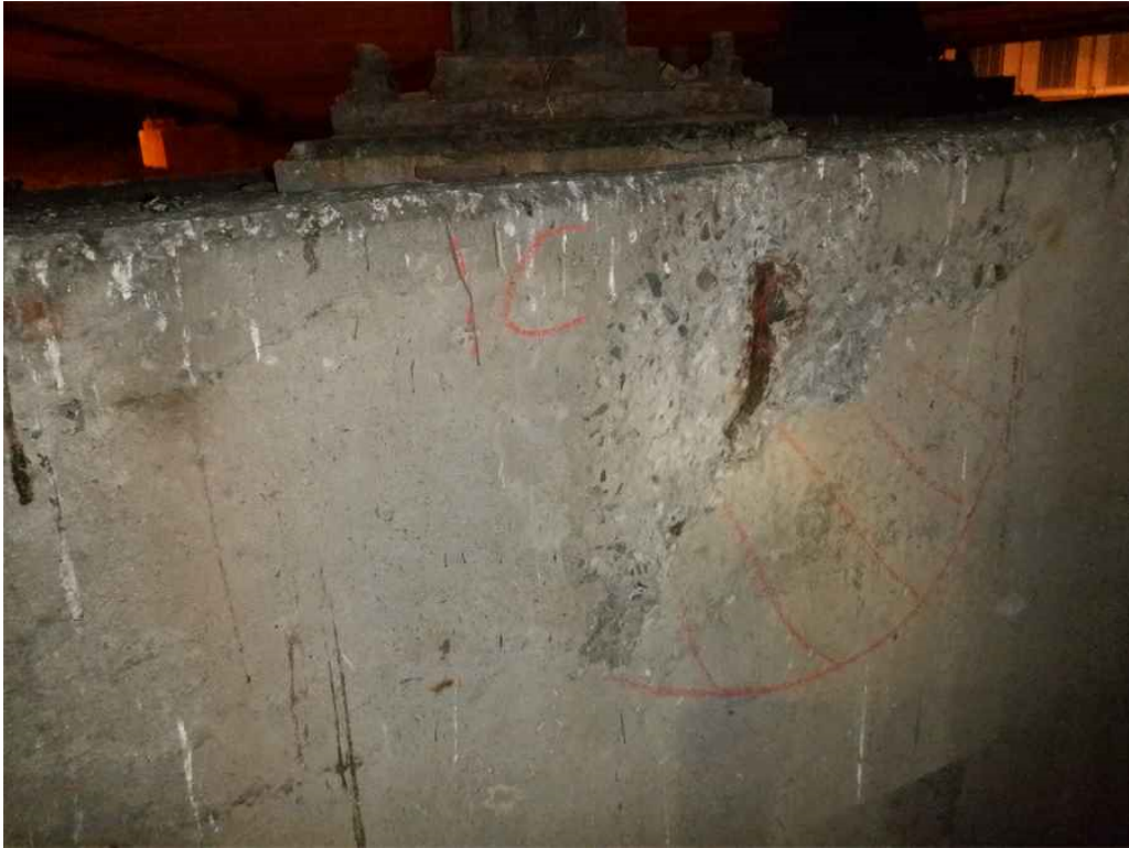
Photo 19: Pier 1 cap, north face, below beam 1C, looking south - spall with exposed rebar and adjacent hollow sounding concrete.
