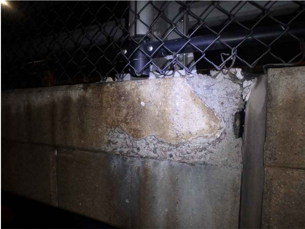
Photo 11: West sidewalk, span 1, at the pier 1 deck joint, looking east - spalling/ heavy scale on the exterior face.
