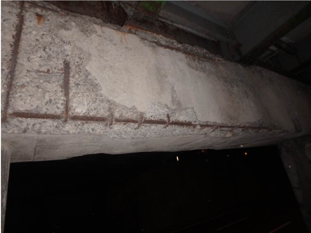
Photo 53: Heavy spalling at pier #1 cap north face bottom corner between Beams C and E (between columns #1 and #2)
