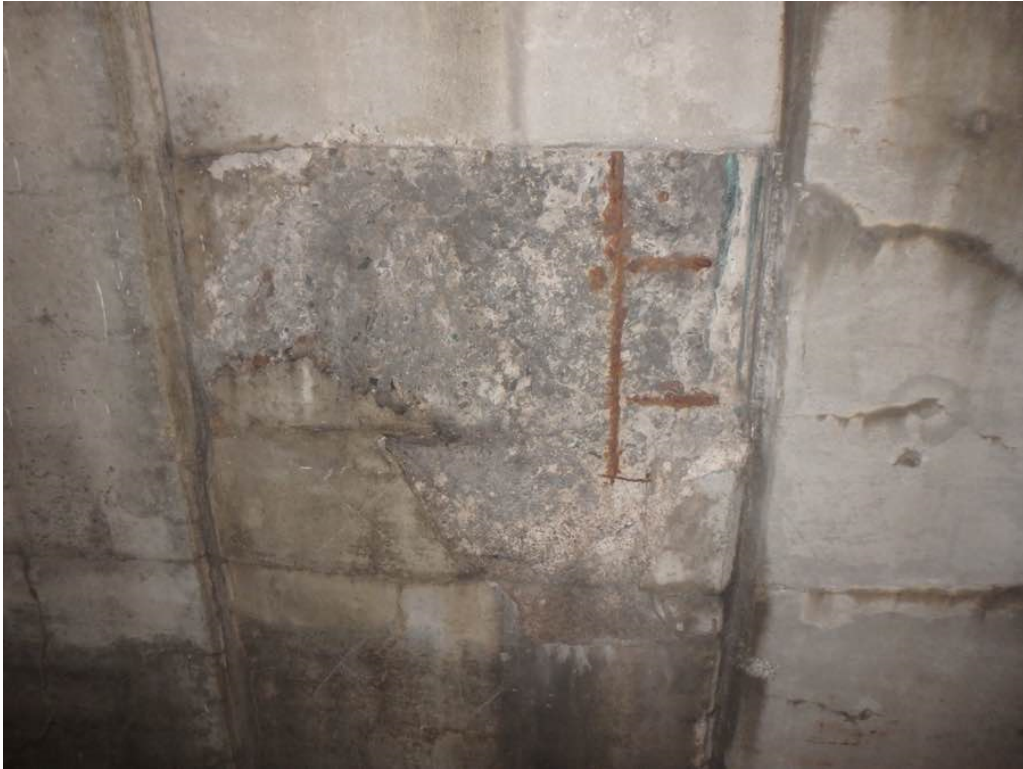
Photo 31: Moderate spalling near the top of the south breastwall below Beam A
