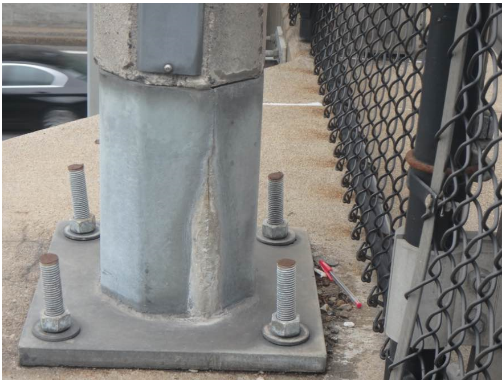
Photo 5: Crack with efflorescence in the east lighting standard in the metal base in span #2 by pier #2
