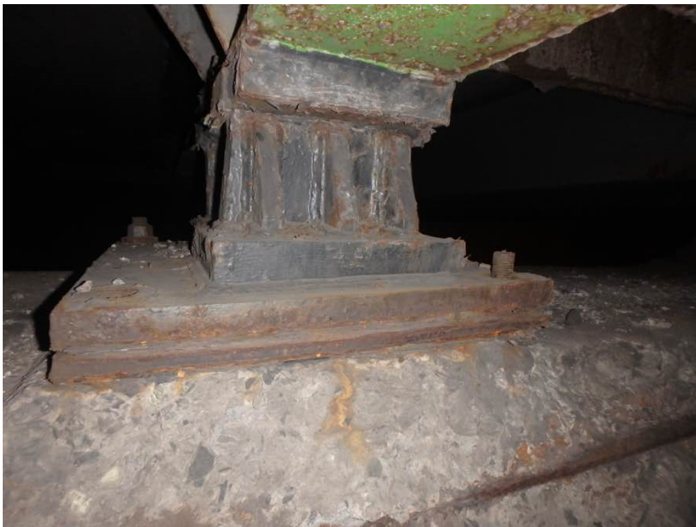
Photo 21: Sheared off anchor bolt and missing anchor nut at Beam E bearing in span #2 at pier #1
