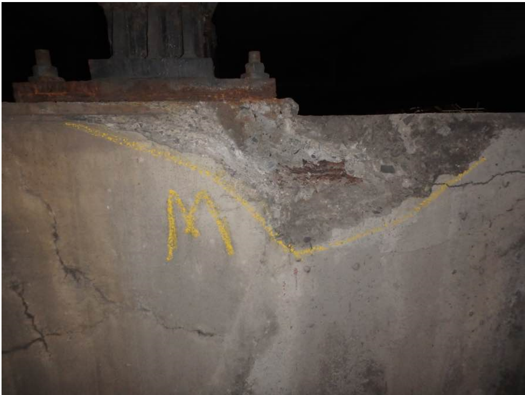
Photo 48: Moderate spalling (no rebar) at the top corner of pier #1 cap south face just east of Beam M
