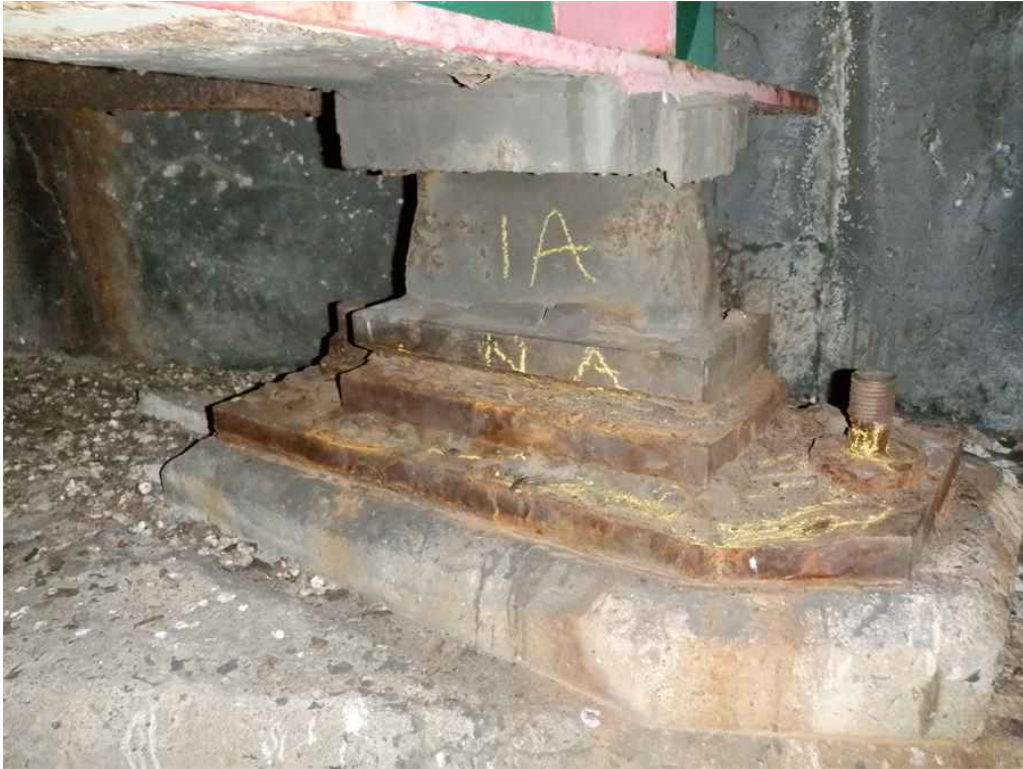
Photo 9: Beam 1A bearing, north abutment, looking north - masonry plate has heavy section loss and anchor bolt nuts have up to 100% section loss.
