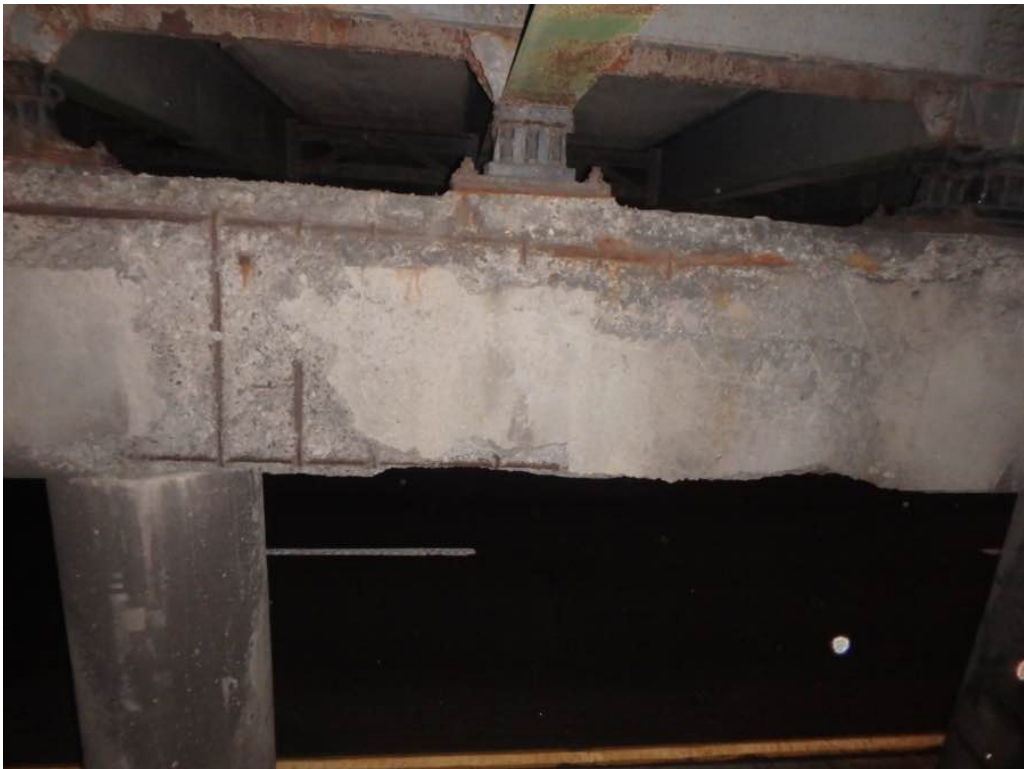
Photo 52: Heavy spalling with exposed rusted rebar and hollow concrete at pier #1 cap north face between Beams C and E
