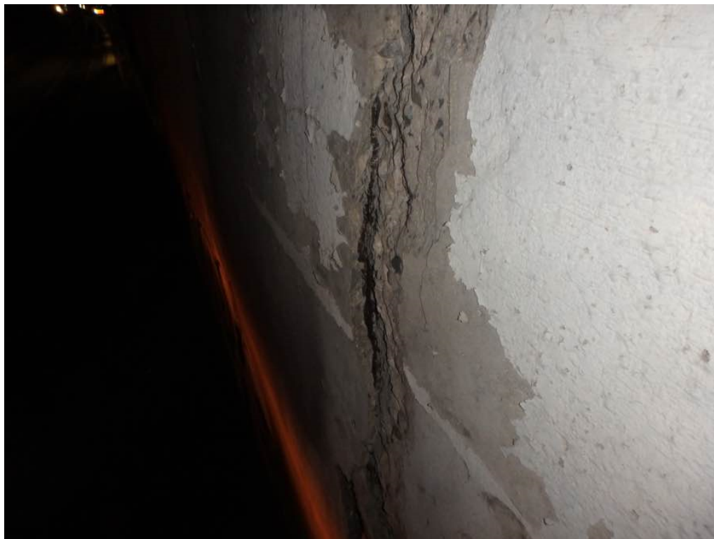
Photo 70: Hollow heavily delaminated concrete on the north face of the pierwall at pier #2 west section between Beams C and E
