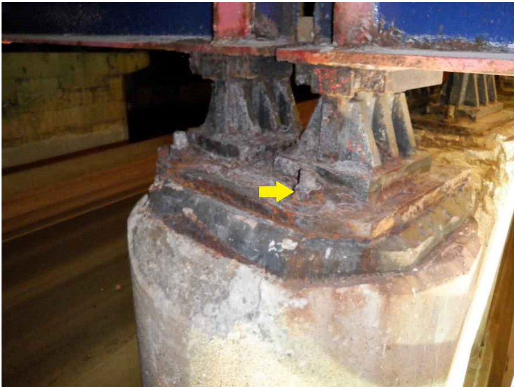
Photo 38: Pier 2 cap, at the west end, at the top, looking northeast - minor scale. Note the southwest anchor bolt nut section loss.
