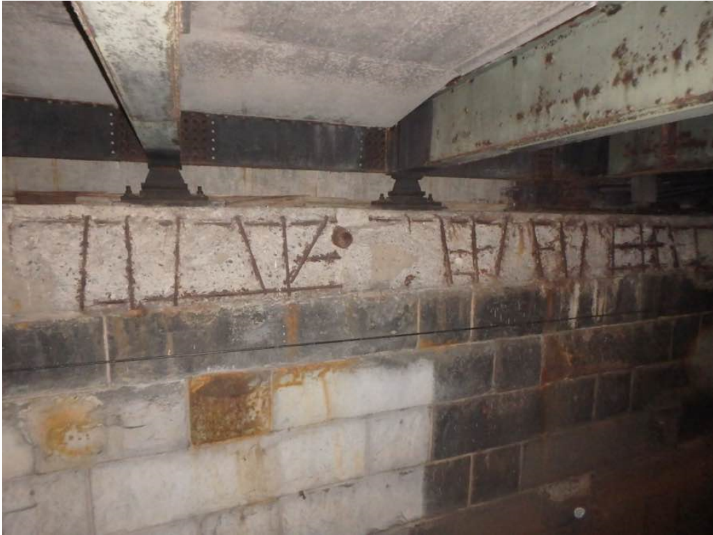
Photo 39: Large spall with exposed rusted and debonded rebar at the north abutment cap between Beams M and P
