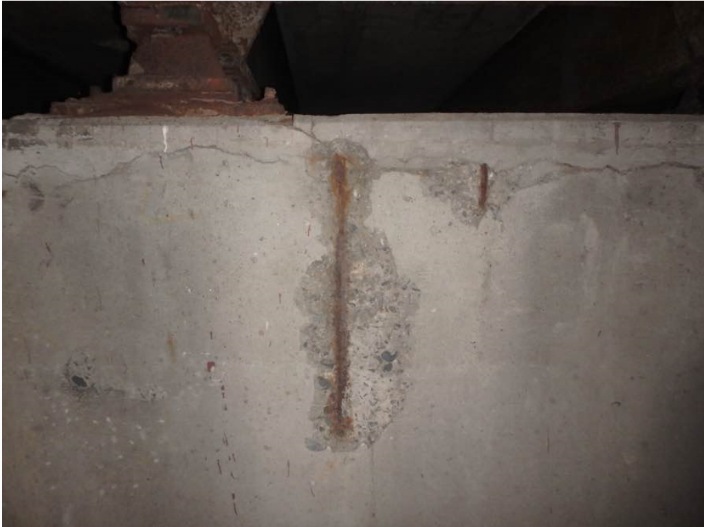
Photo 67: Moderate spalling with exposed rusted rebar and horizontal cracking at the top and an area of minor hollow concrete with edge spalling at pier #2 cap north face between Beams K and L
