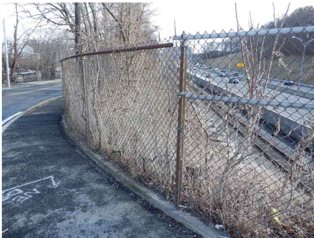
Photo 45: Northeast approach guardrail, second post from the north abutment, looking east - top rail is disconnected.
