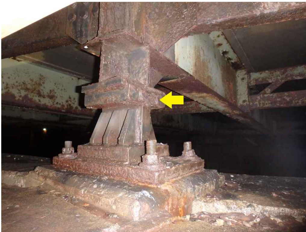
Photo 22: Same location as the previous photo, looking northwest - the east keeper plate is missing.
