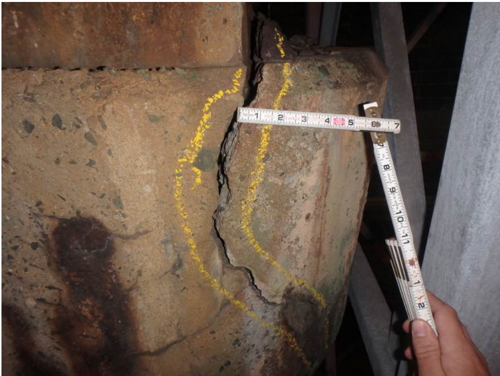
Photo 62: Heavy crack and delaminated concrete on the south face of pier #2 cap at the east end
