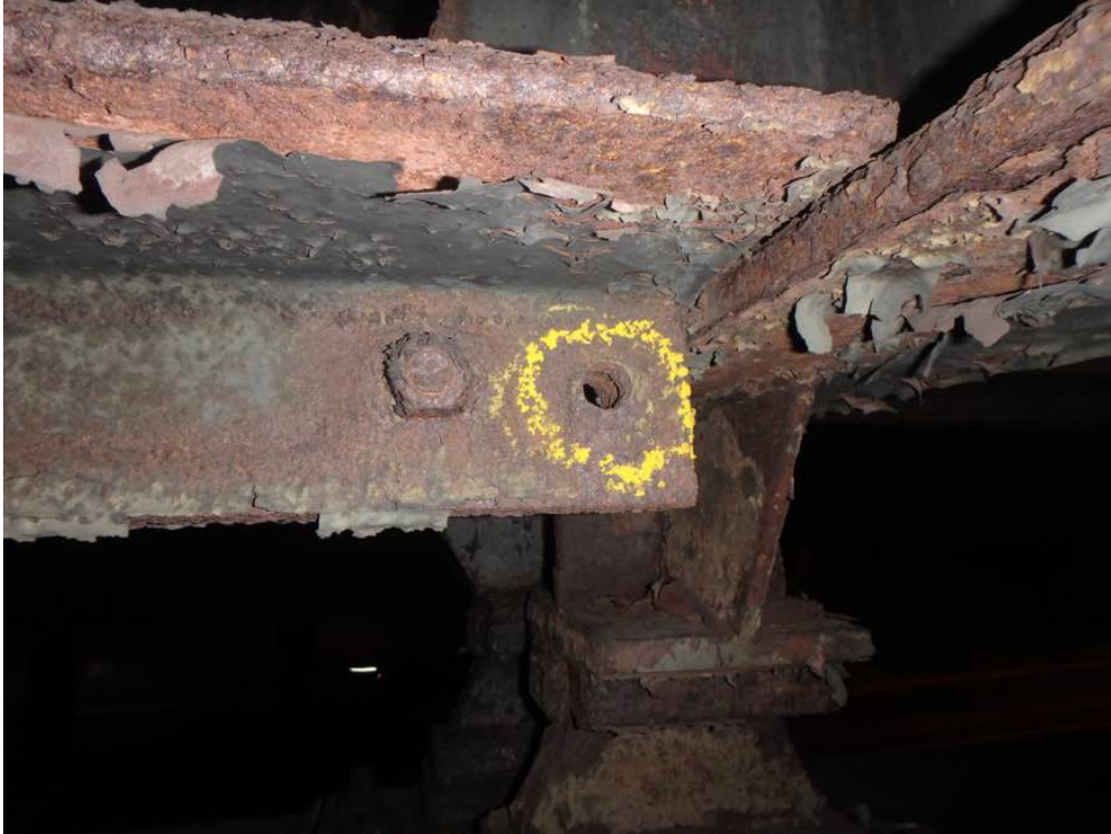
Photo 24: Missing bolted connection at the first utility support in bay #6 in span #3 adjacent to Beam F
