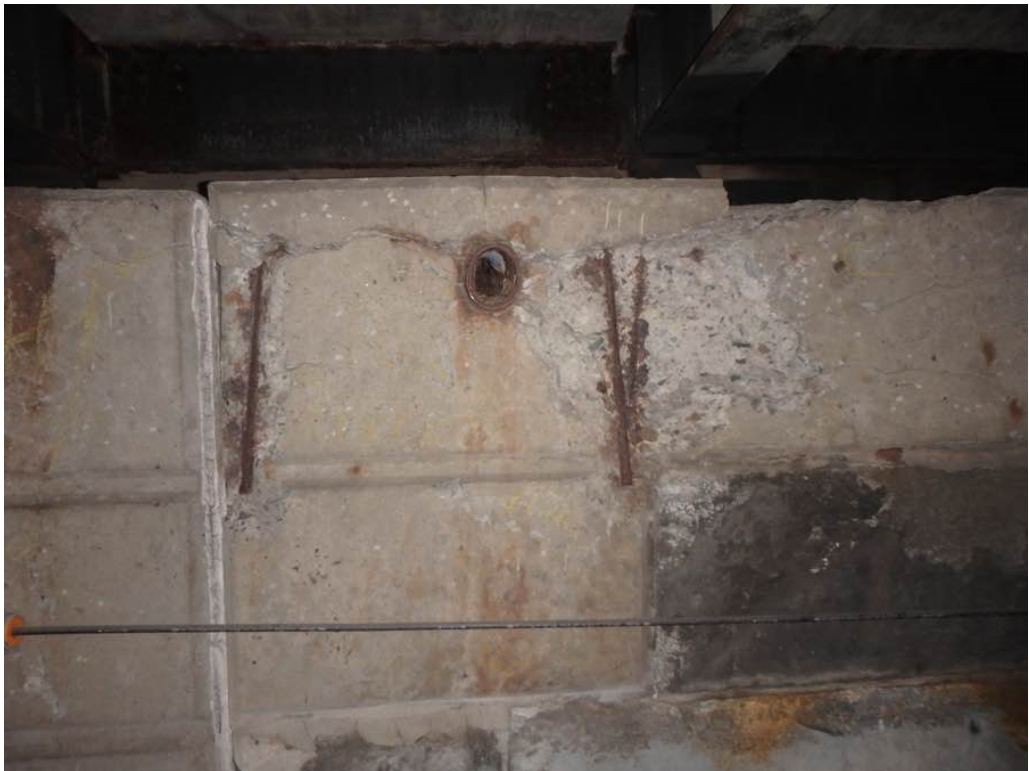
Photo 36: Moderate to heavy spalling with exposed rusted rebar, hollow concrete, and horizontal cracking at the top of the north breastwall between Beams D and E
