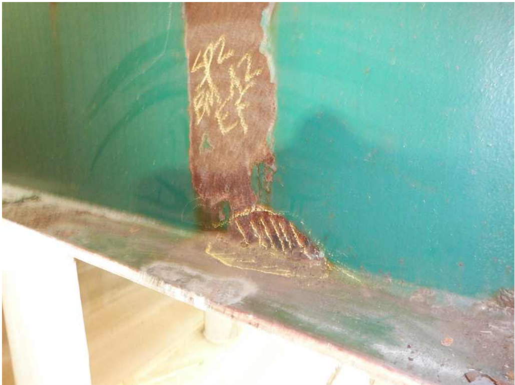
Photo 18: Beam 2A, span 2, east web above the left dashed white line, looking west - isolated area moderate rust with section loss.
