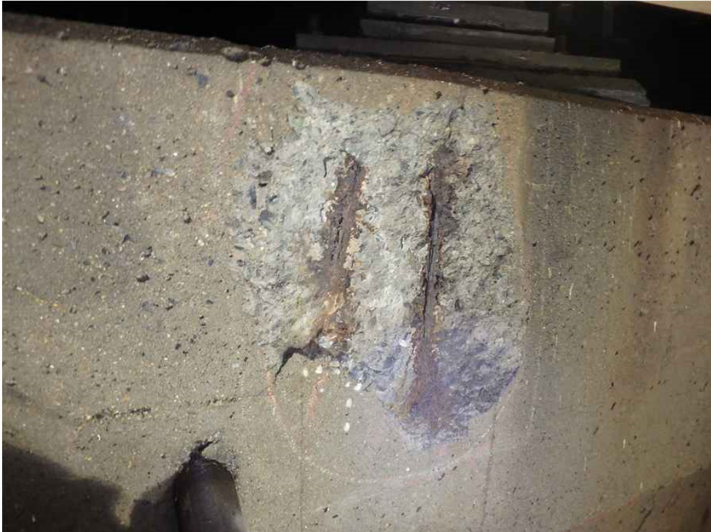
Photo 31: Pier 1 cap, south face below beam 2C, near the top, looking north - spall with exposed rebar and surrounding hollow area.
