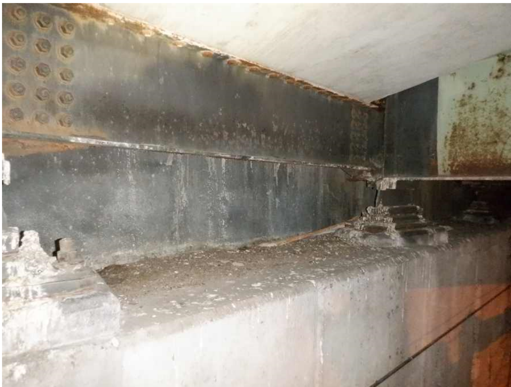
Photo 14: North abutment bridge seat, between beams 1C and 1D - moderate debris and pigeon droppings scattered throughout.
