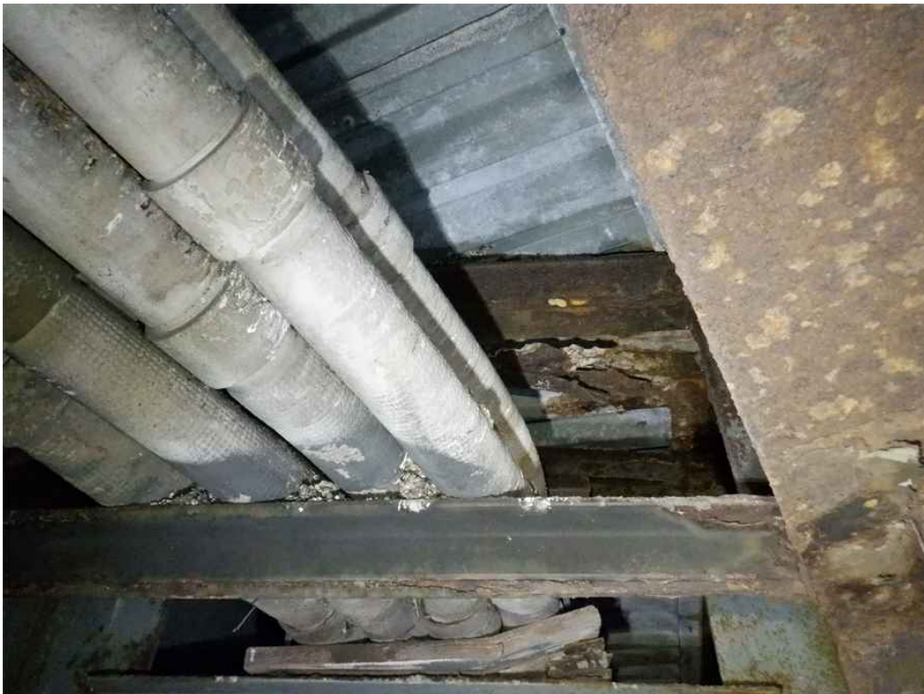
Photo 4: Stay-in-place form, span 1, bay 1, near pier 1, behind end diaphragms - an area of heavy rust with severe corrosion.
