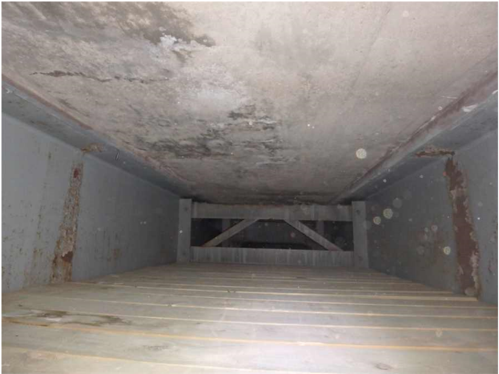
Photo 9: Underside of deck, span 3, bay 5, near the north 1/4 point, looking north - longitudinal and transverse cracks with light efflorescence and moisture stains.
