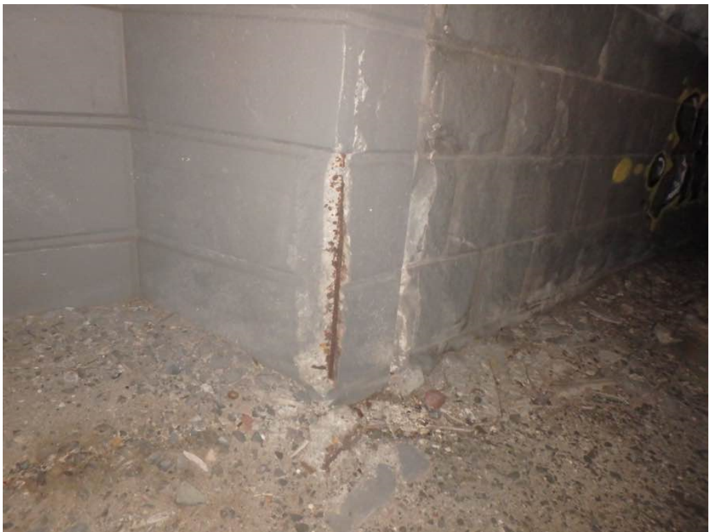
Photo 35: Moderate spall at the bottom of the north breastwall just east of Beam D
