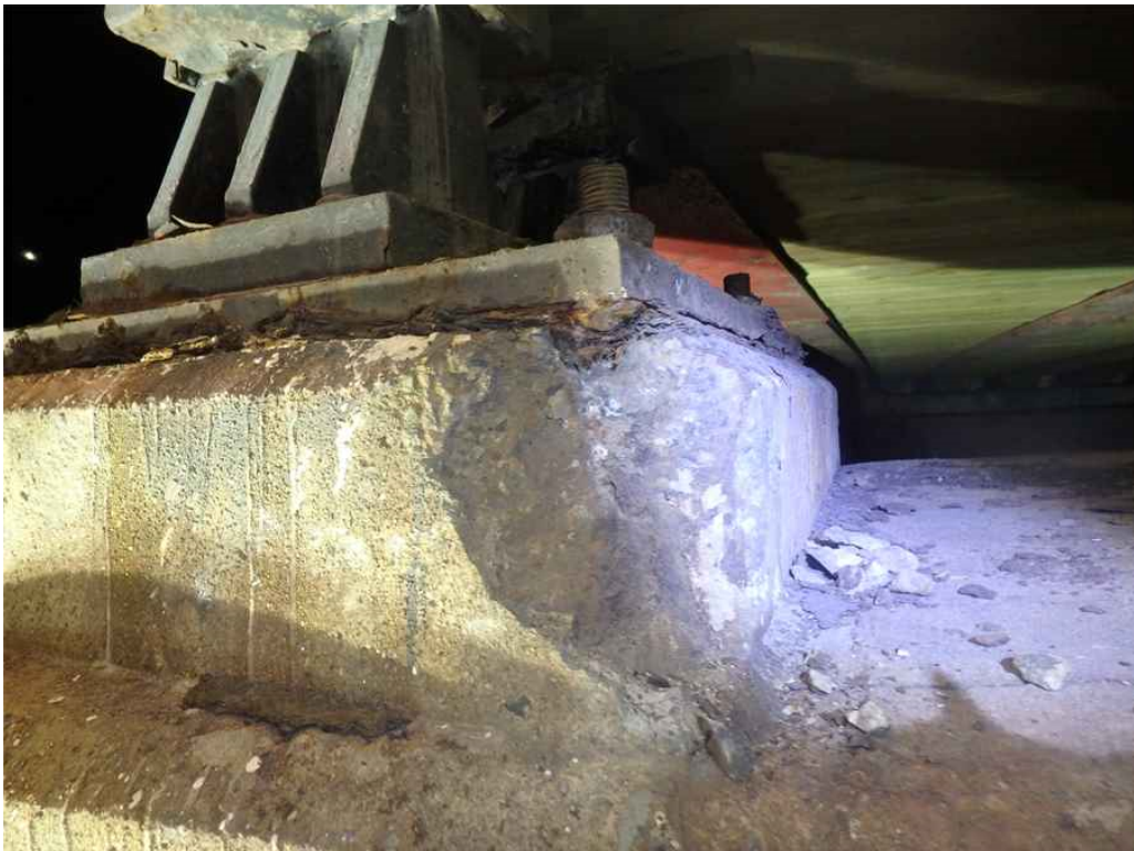
Photo 24: Beam 2A bearing, span 2 at pier 2, looking southeast - spall in the northwest corner of the pedestal that slightly undermines the bearing.
