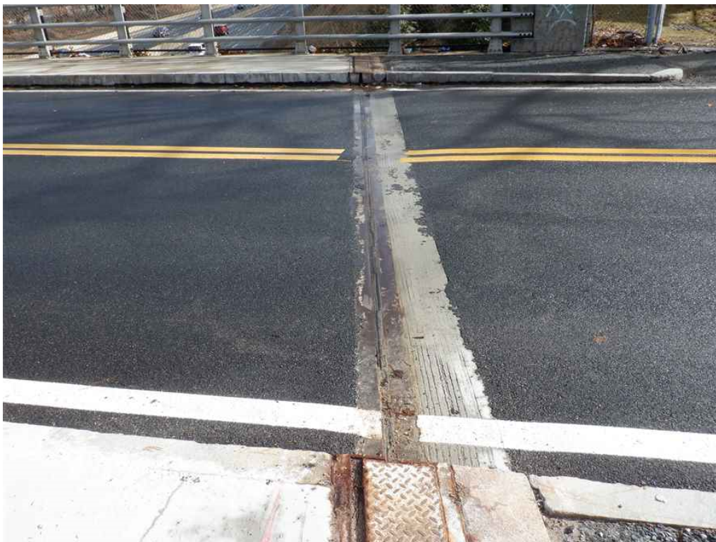
Photo 14: South abutment deck joint, looking east - previously noted deficiencies have been repaired.
