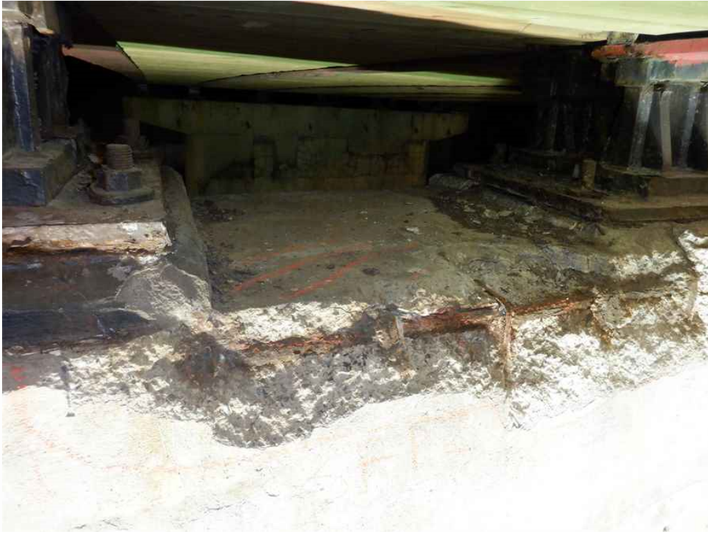
Photo 37: Pier 2 cap, south face between beams 3F and 3G, at the top, looking north - spall with exposed and debonded rebar.
