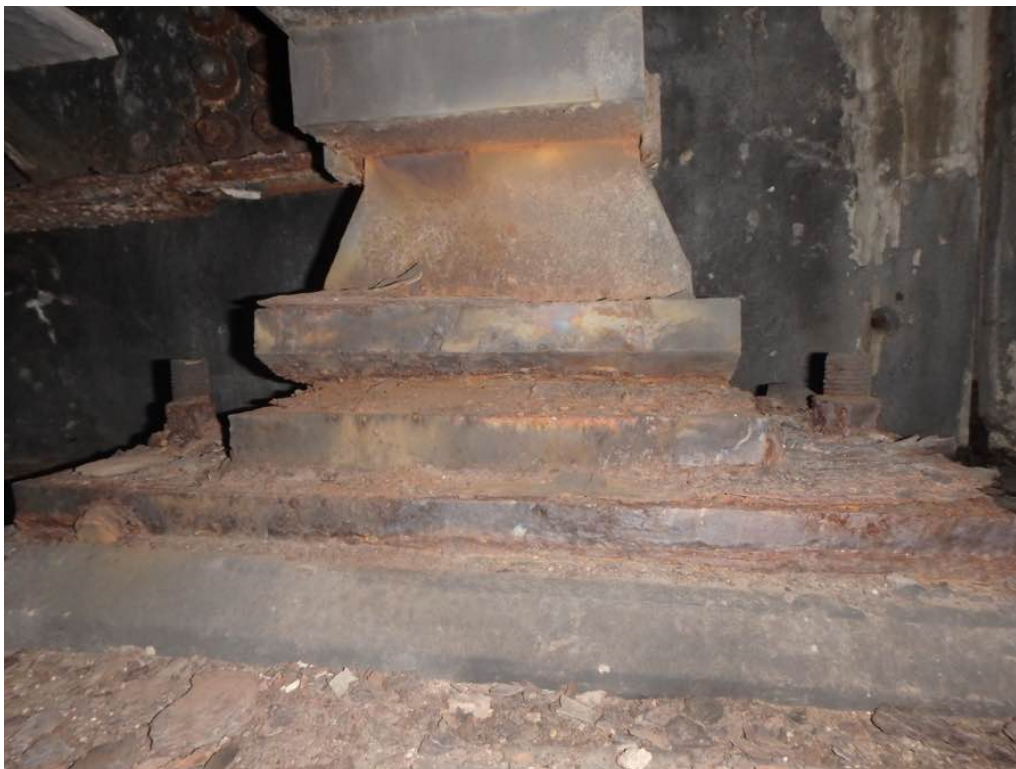
Photo 22: Impacted rust between the rocker and masonry plate at Beam H at the north abutment
