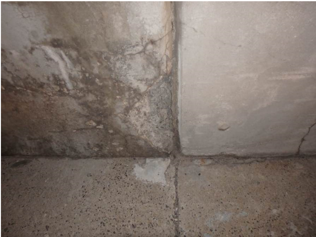
Photo 30: Moderate spalling at the bottom of the south breastwall outside Beam A
