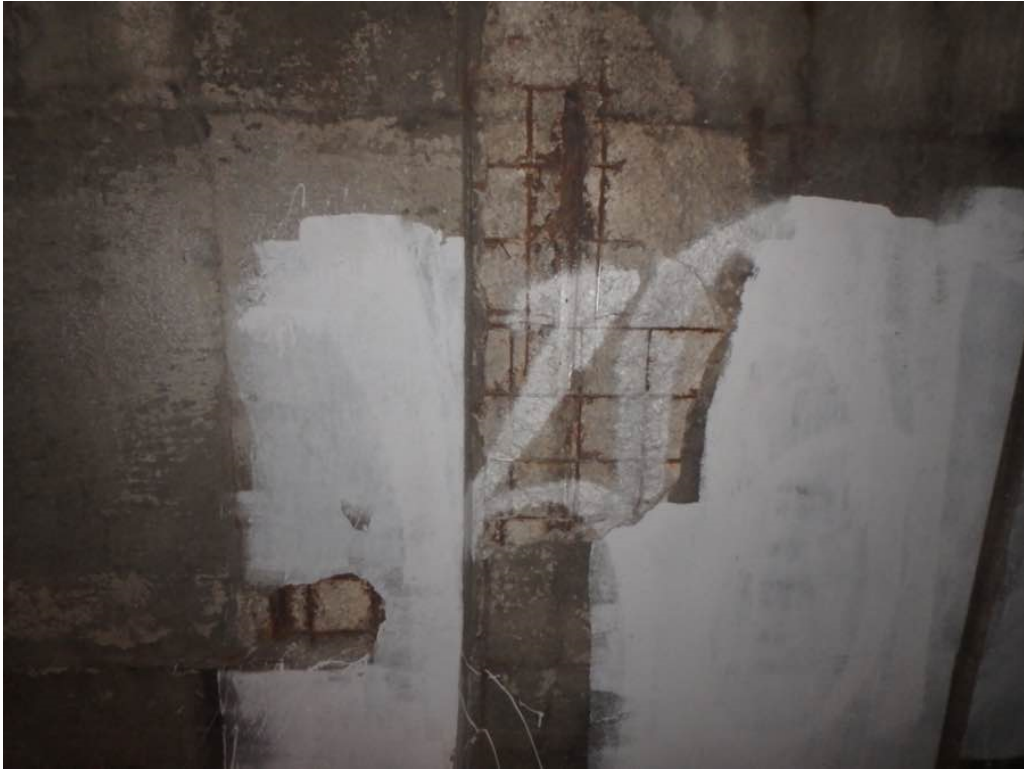
Photo 33: Moderate spalling with delamination and hollow concrete at mid-height at the south breastwall below Beam M
