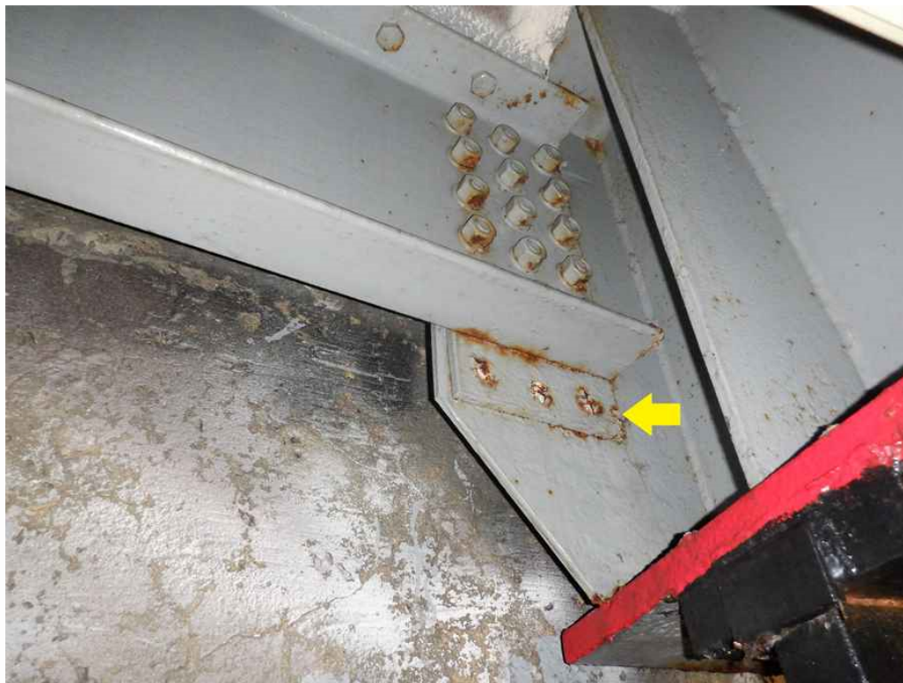
Photo 19: End diaphragm, bay B, at the east face of beam 3C, looking south - the bottom connection bolts are missing.
