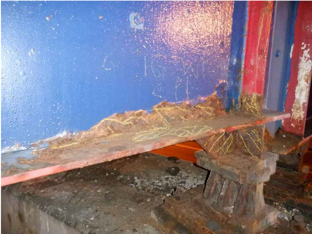
Photo 8: Beam 1G, span 1, at pier 1, looking southeast - web and bottom flange has section loss.
