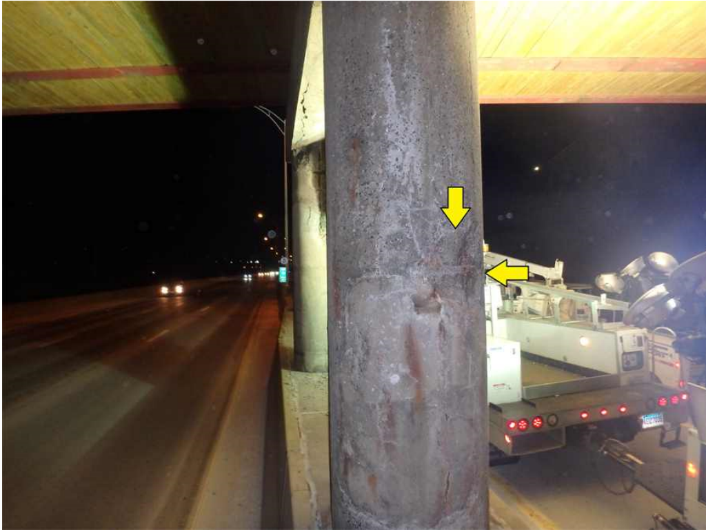
Photo 41: Pier 2, column 2, looking east - the west face of the column has a spall with exposed rebar and surrounding hollow areas.
