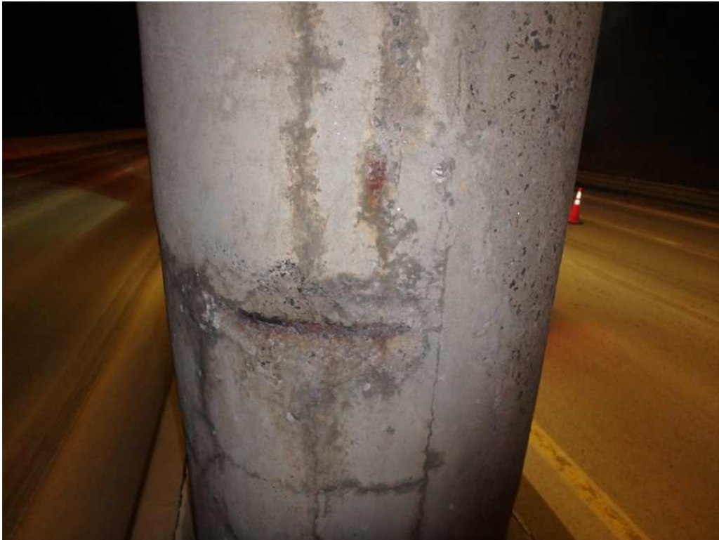
Photo 42: Pier 2, column 3, looking east - the west face of the column has a spall with exposed rebar.
