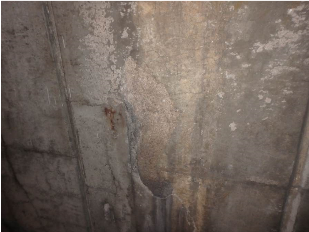
Photo 34: Moderate spall near the bottom of the south breastwall below Beam R
