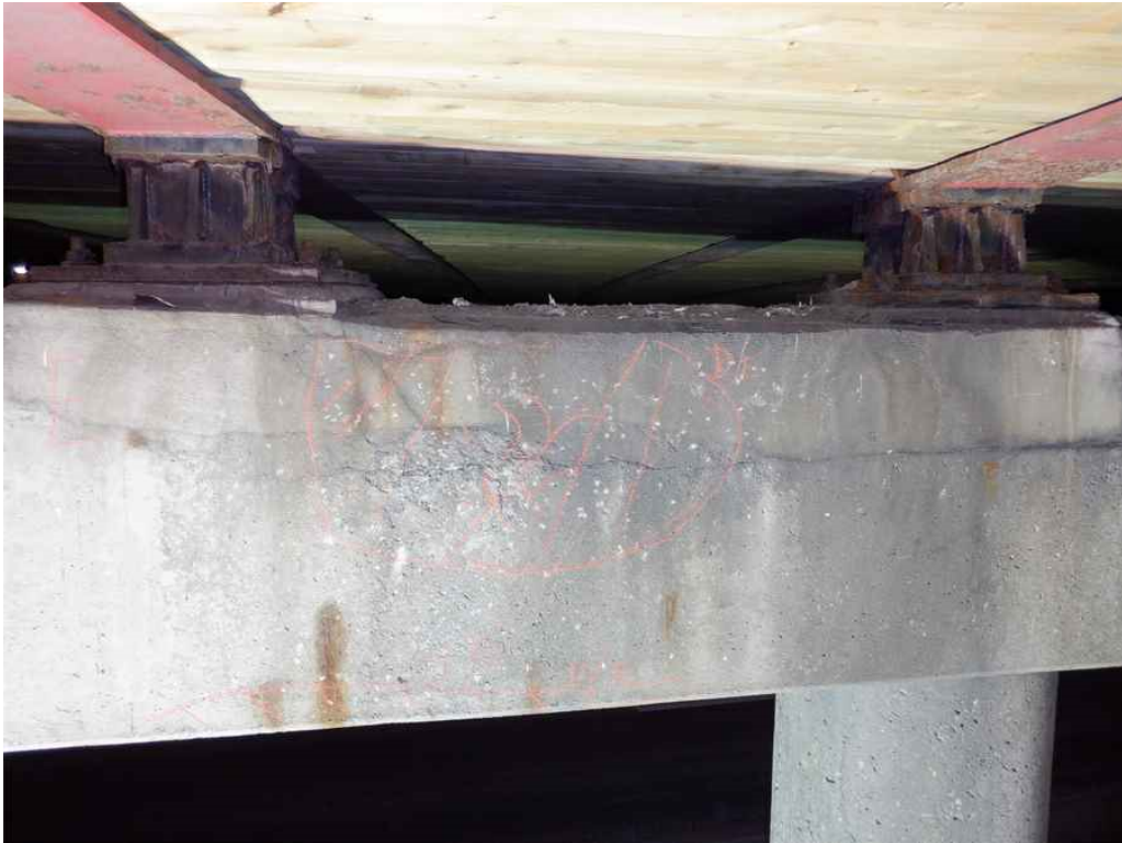
Photo 36: Pier 2 cap, south face between beams 3D and 3E, looking north - there are cracked hollow areas at the top and bottom.
