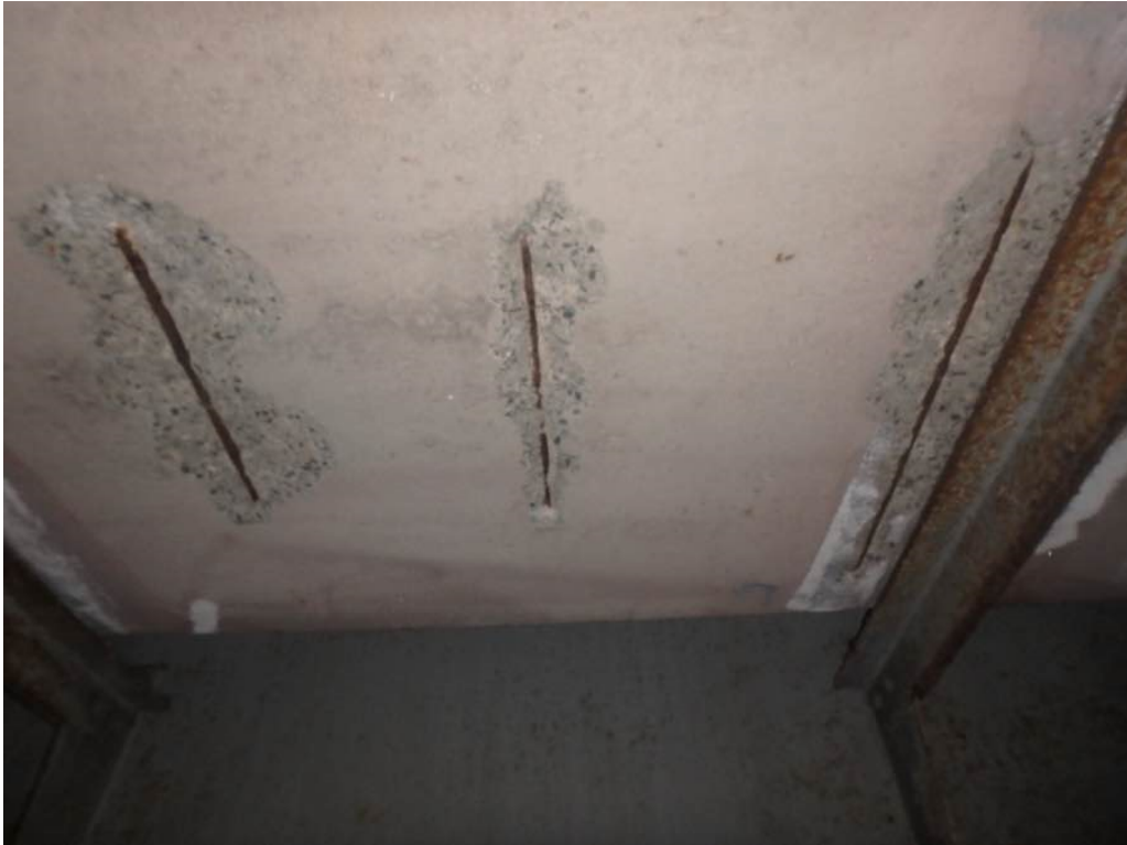
Photo 13: Three minor spalls on the bottom face of the concrete encased utility duct in bay #2 in span #2 between the fifth and sixth utility supports from pier #1 (above the second travel lane)
