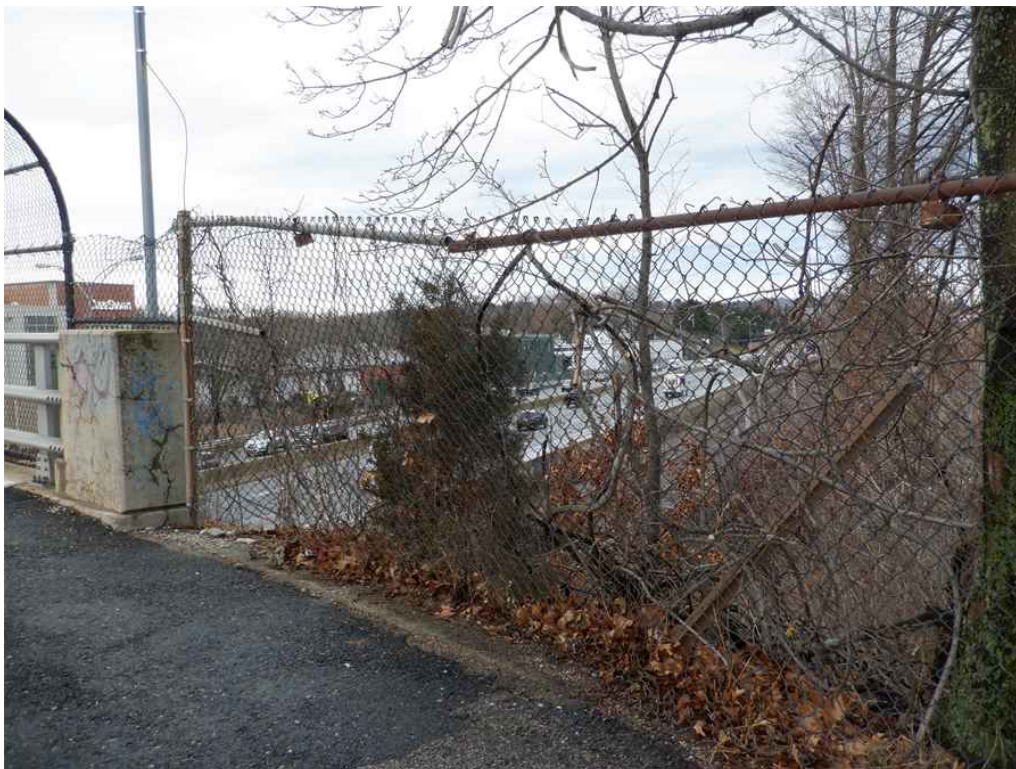
Photo 44: Northwest approach guardrail, looking southwest - the second post is missing and the third post is detached. Note the sagging fence.
