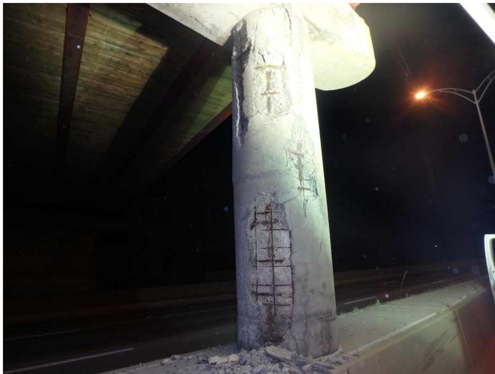
Photo 40: Pier 2, column 1, looking northeast - the south and west faces of the column are heavily deteriorated.
