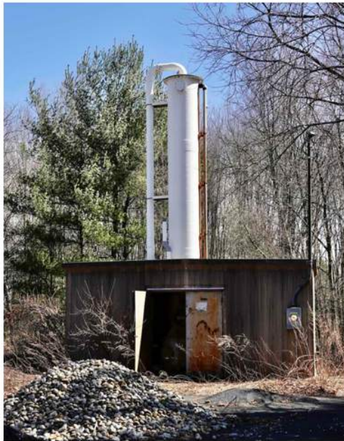
Facility installed behind Shaw's Plaza to remove trichloroethylene (TCE) from the groundwater
