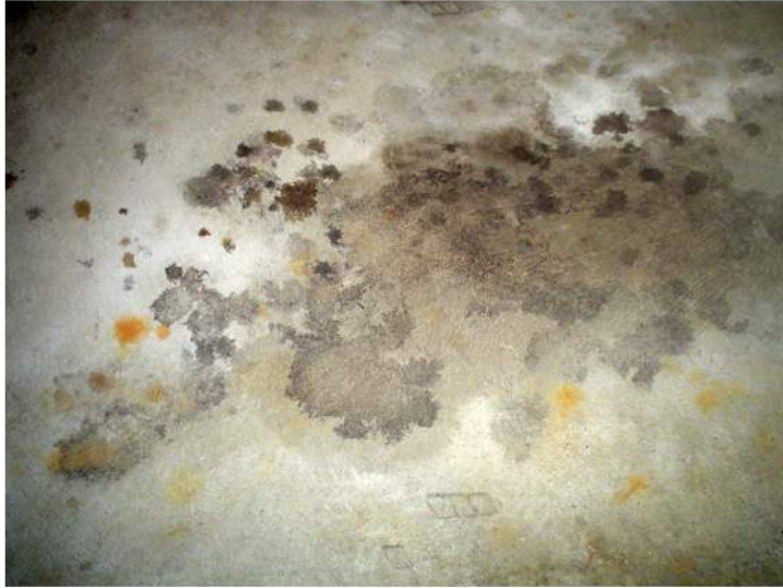
Automotive chemicals stained this garage floor.
