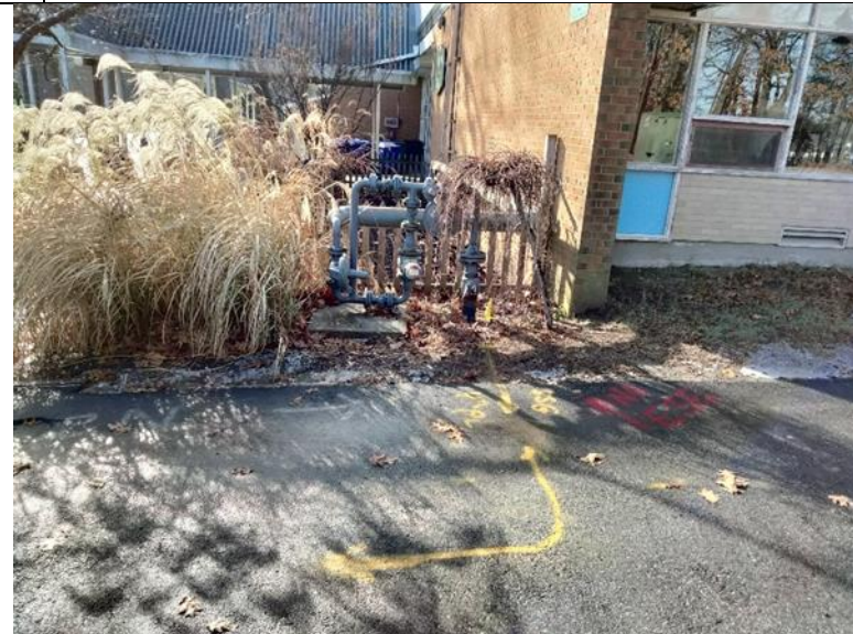
Photo #8: Natural gas pipes at the northeast corner of the school
