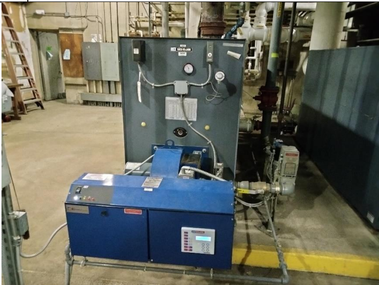
Photo #11: Natural gas boilers
