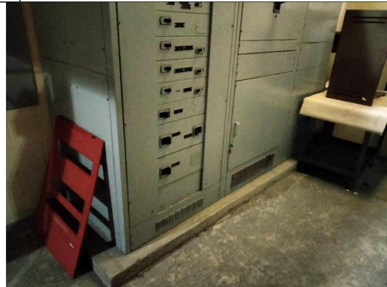
Photo #16: Electricity service room
