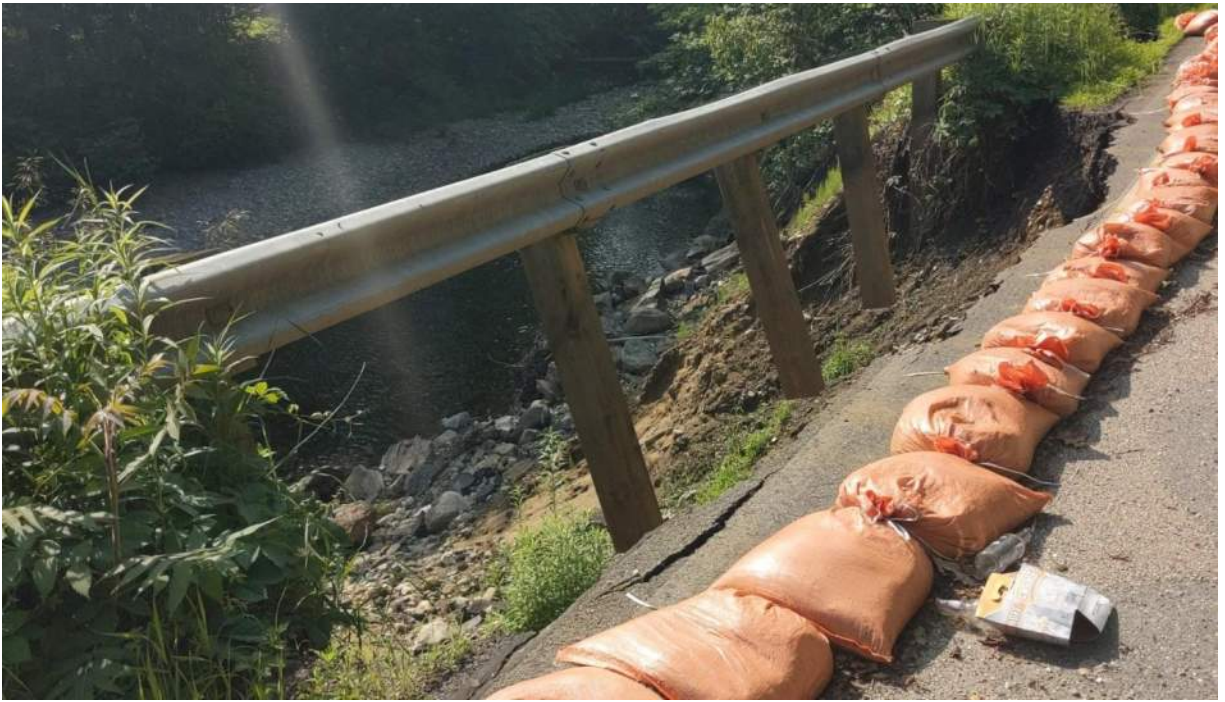
Photo #3: Another view of the collapsed embankment. The soil around the posts of the guardrails is completely gone. Facing southeast.
