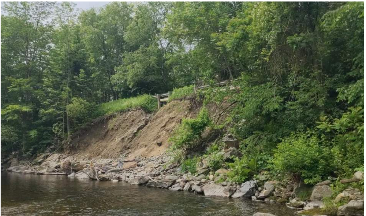
Photo #8: View of the entire exposed area resulting from the embankment failure. Facing south.
