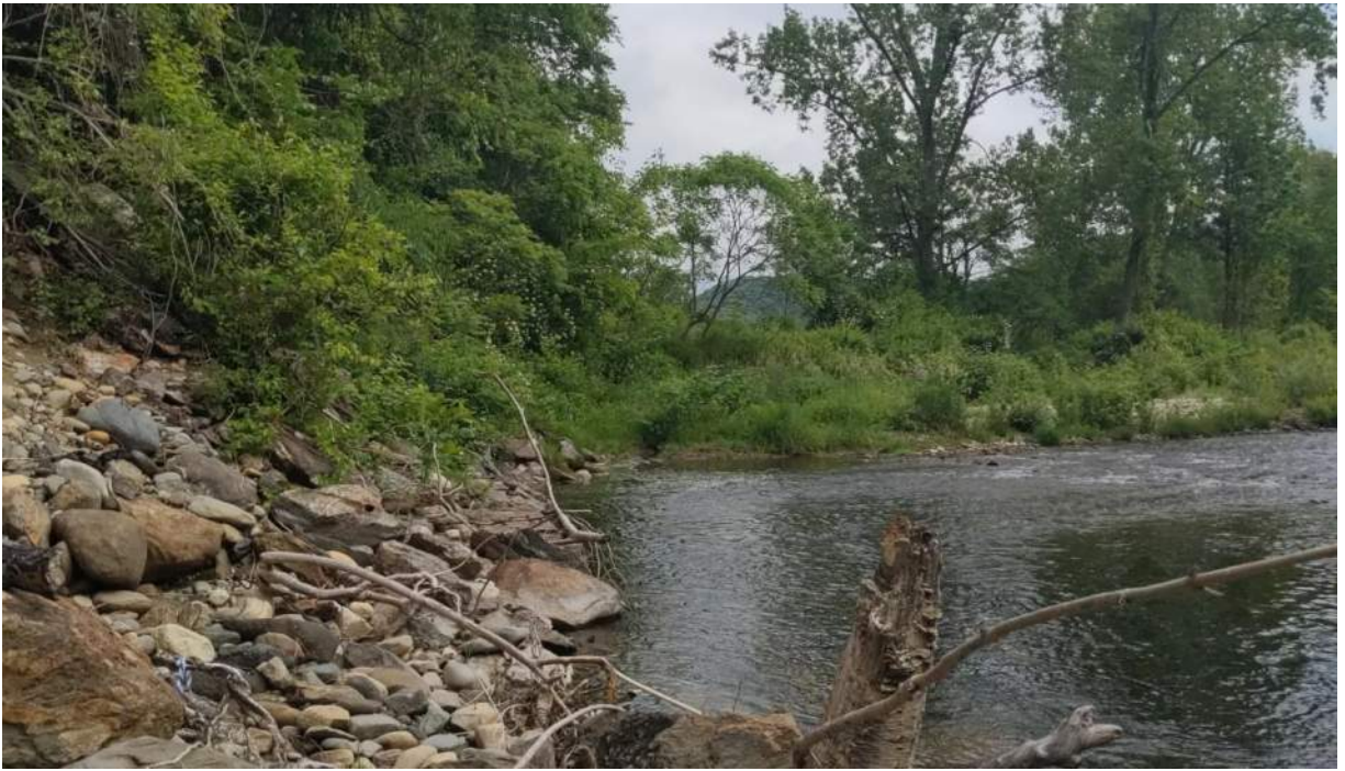
Photo #5: View of the embankment upstream of the collapsed section. Facing north.
