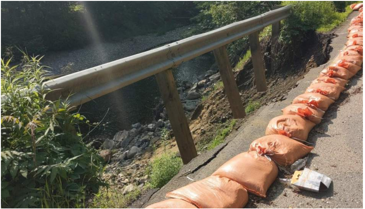
Photo #3: Another view of the collapsed embankment. The soil around the posts of the guardrails is completely gone. Facing southeast.
