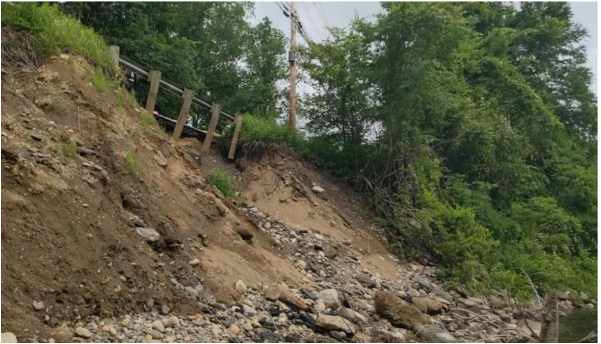
Photo #9: View of the exposed area resulting from the embankment failure. Facing northwest.
