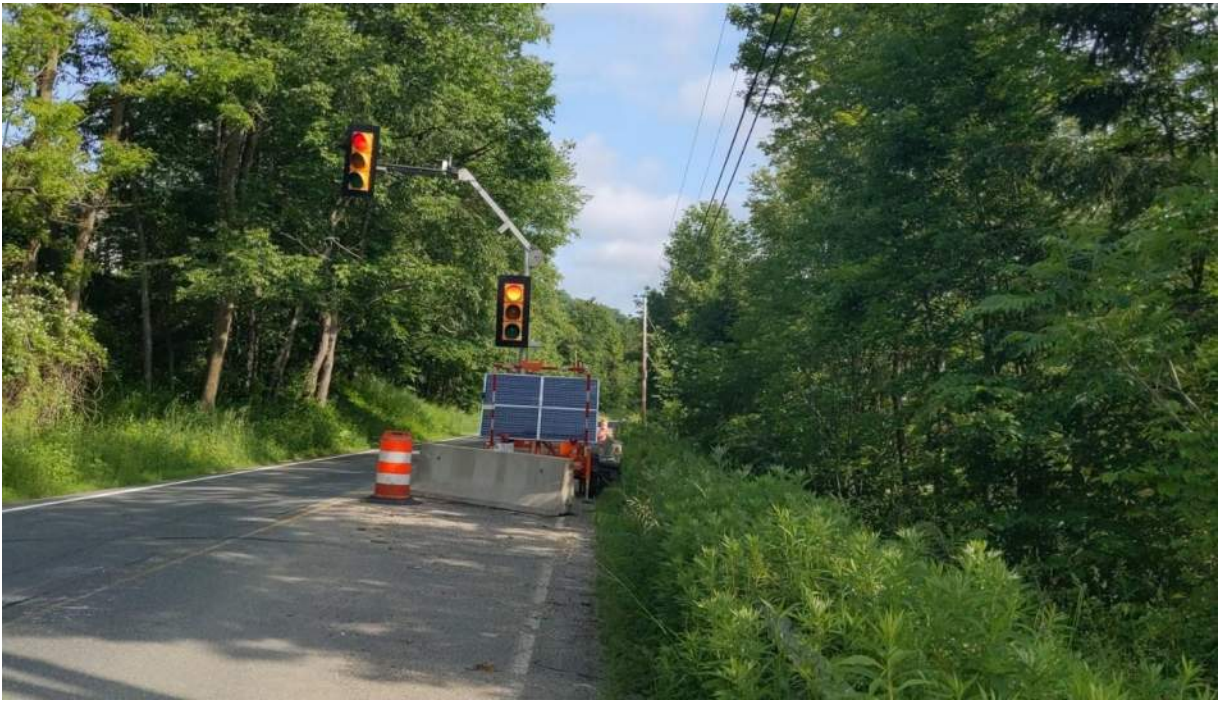
Photo #1: View of the Jacksonville Road which has one lane closed as a result of the embankment failure. Facing northwest.
