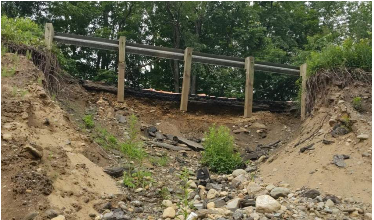
Photo #4: View of the collapsed embankment from below. Facing west.
