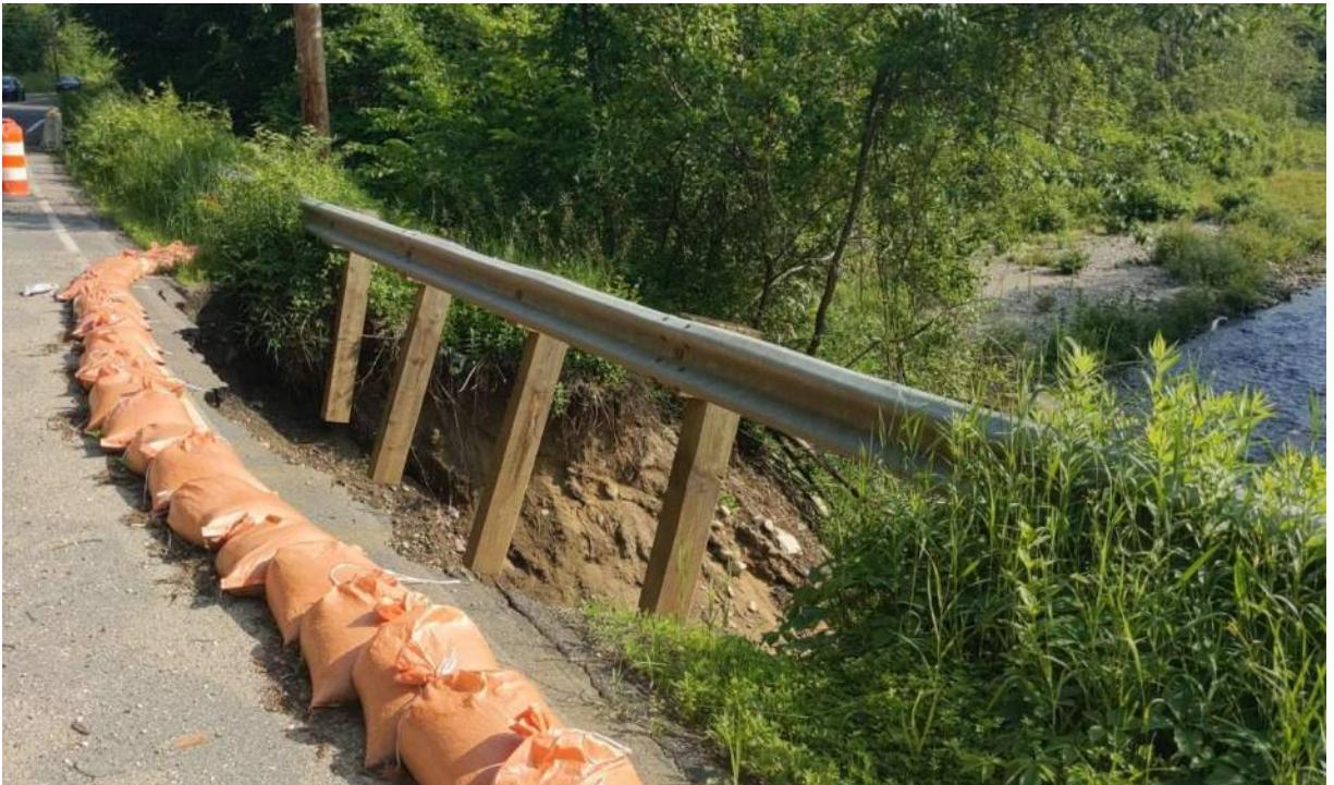
Photo #2: View of the collapsed section of the embankment. Facing north.
