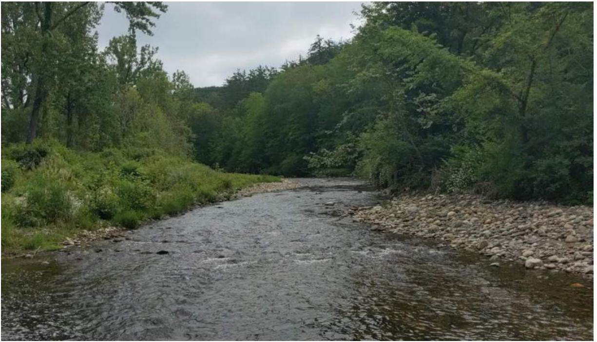
Photo #7: View of the river upstream of the collapsed section of the embankment. Facing northeast.
