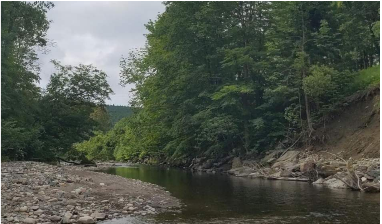
Photo #6: View of the embankment downstream of the collapsed section. Facing southeast.
