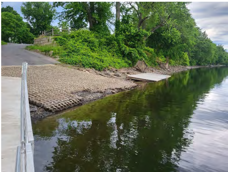
Image of boat ramp, taken standing on floating dock, looking north/upstream. Photo shows edge of ramp blocks falling away as well as area where fill will need to be added and pilings to secure upstream dock.
