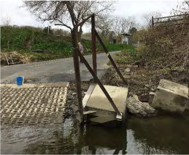
Concrete debris and remnant piling from former dock structure. To be removed.
