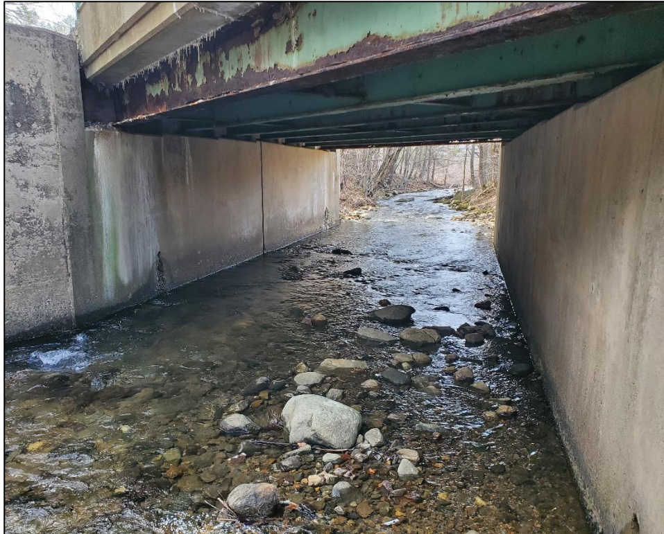
Photo 3. Potter Brook beneath bridge/Cyrus Stage Road showing proposed impact area View south (downstream)
