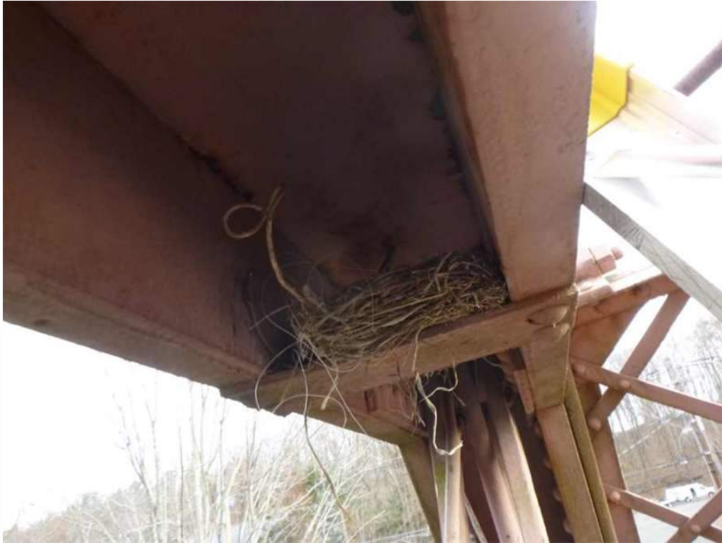
Photo 61: Bird's nest sitting on batten plates near Panel Point U8.
