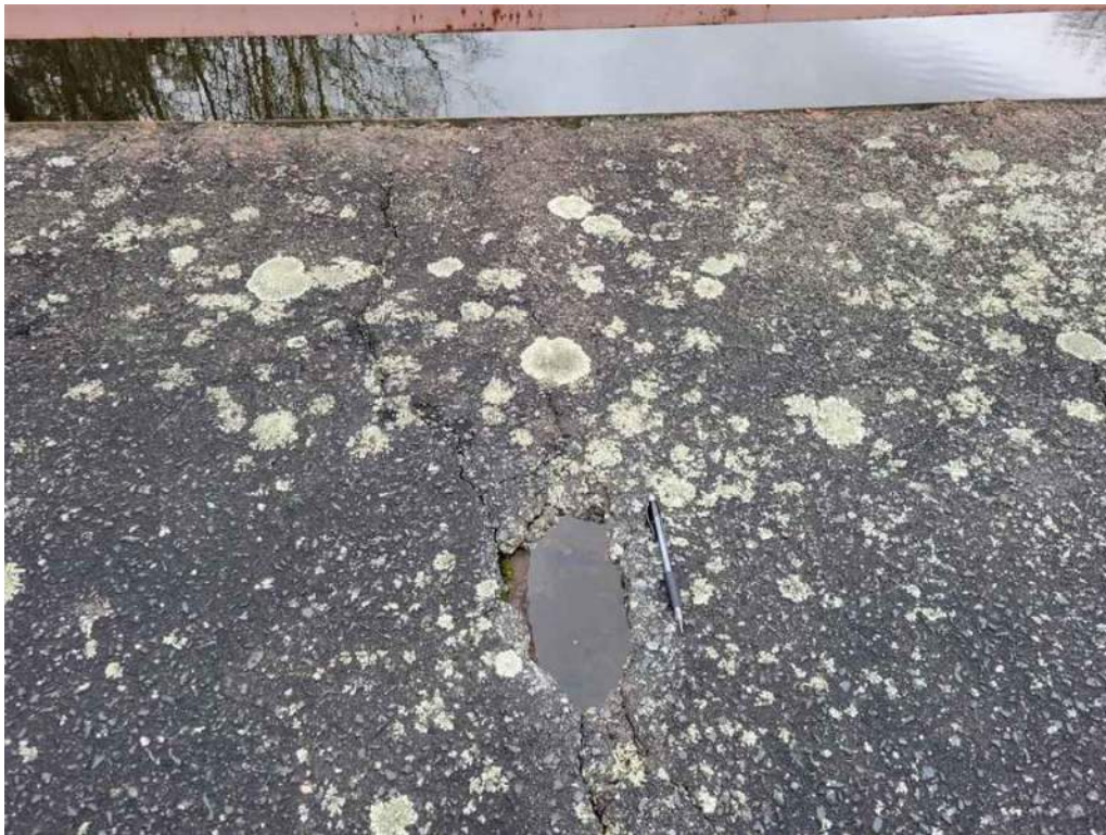
Photo 16: 30" from the north side, 10" wide x 4" long hole with 100% section loss to the deck, 102" to the east of Floorbeam 3.
