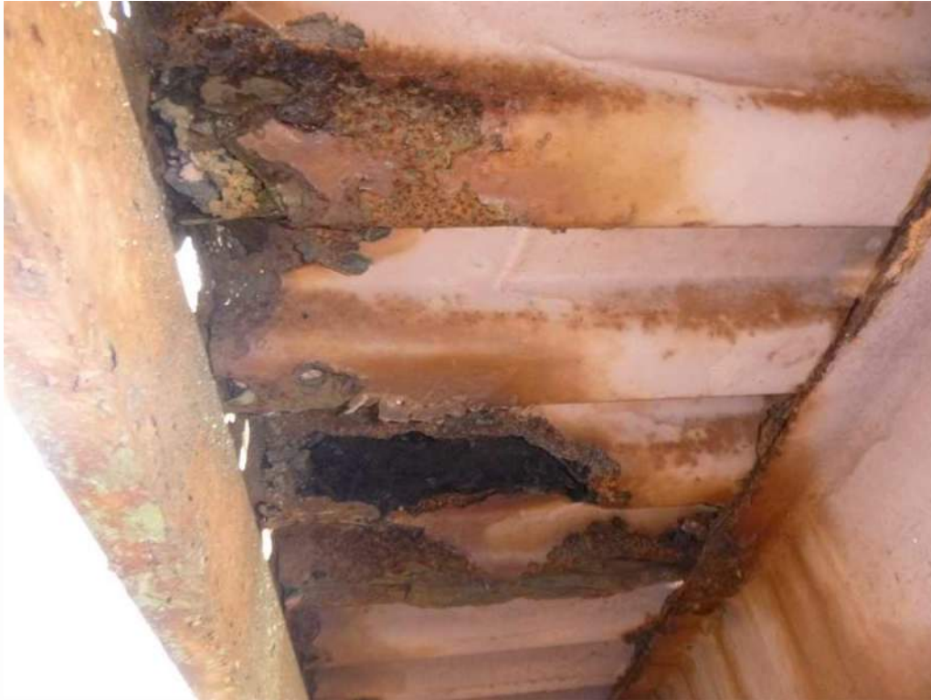
Photo 23: Bay 5, north overhang, three (3) 1'-0" wide holes, 100% section loss to bottom of corrugated steel deck.
