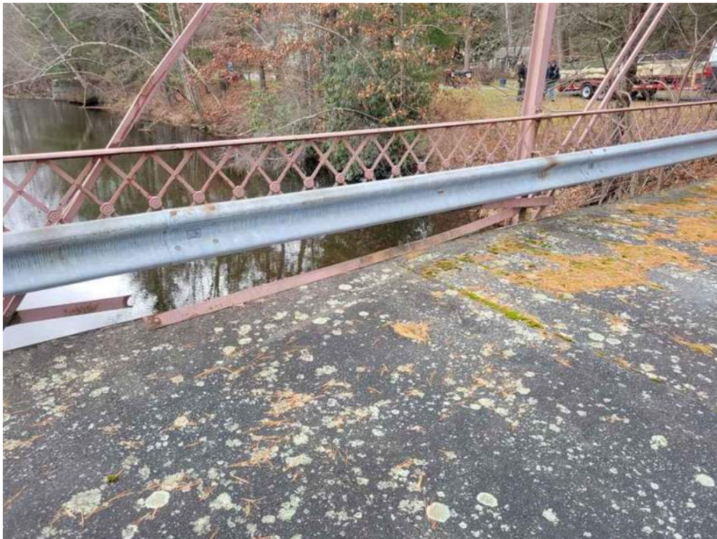
Photo 36: On the south truss, at Panel Point L2 the bottom horizontal bar is unattached from the railing at one end.
