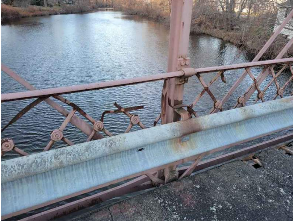
Photo 33: On the north truss, at Panel Point 5, the cross bracing is deformed and rusting.
