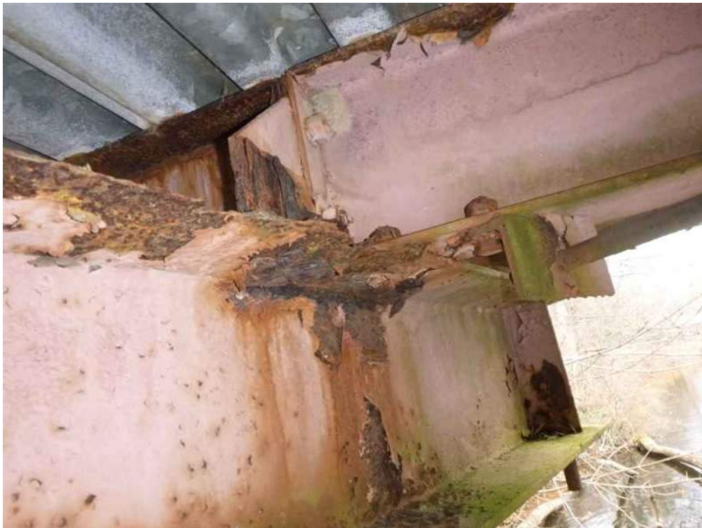
Photo 2: 100% loss of section to the top flange of Floorbeam 1 at Stringer 4.
