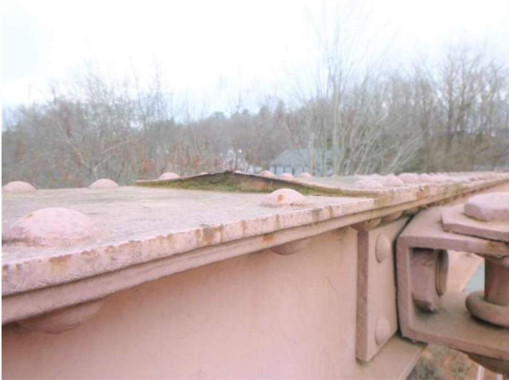
Photo 59: There is up to 2" of pack rust between the top plate and the cover plate at Panel Point U7.
