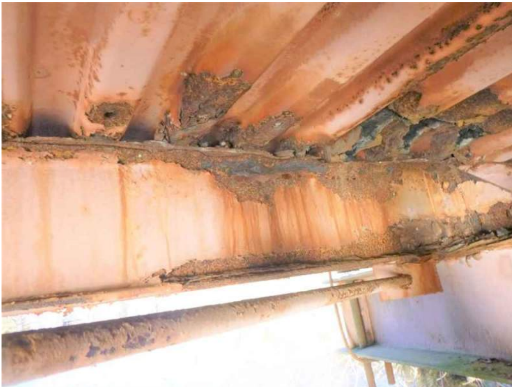
Photo 46: Bay 7, Stringer 4 at Floorbeam 7 there is 100% loss of section to top flange and web of Stringer 4.
