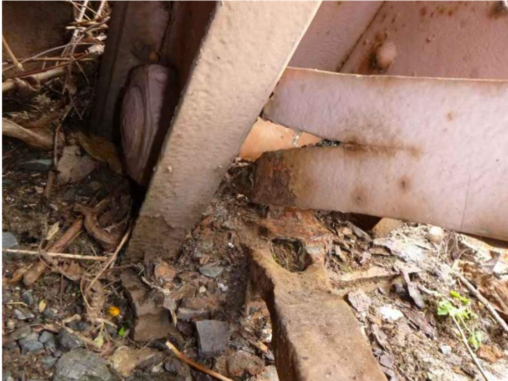
Photo 63: At the east abutment, north truss, Member L9 exhibits up to 10% section loss to the end of the exterior lower chord eye bar.
