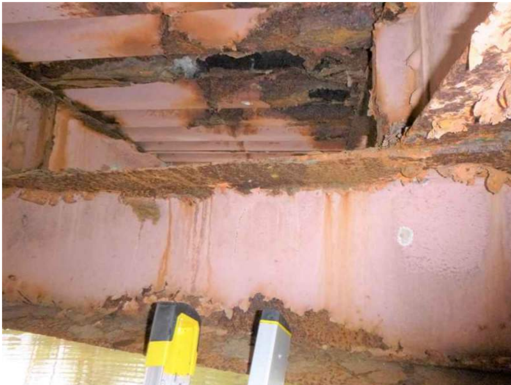
Photo 54: Up to 1/4" loss of section to the top flange of Floorbeam 7 between Stringers 2 and 3.
