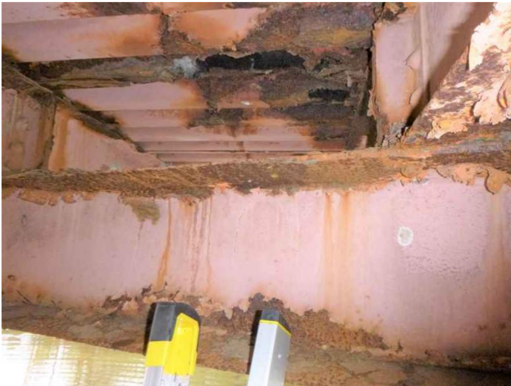
Photo 6: Up to 1/4" loss of section to the top flange of Floorbeam 7 between Stringers 2 and 3.
