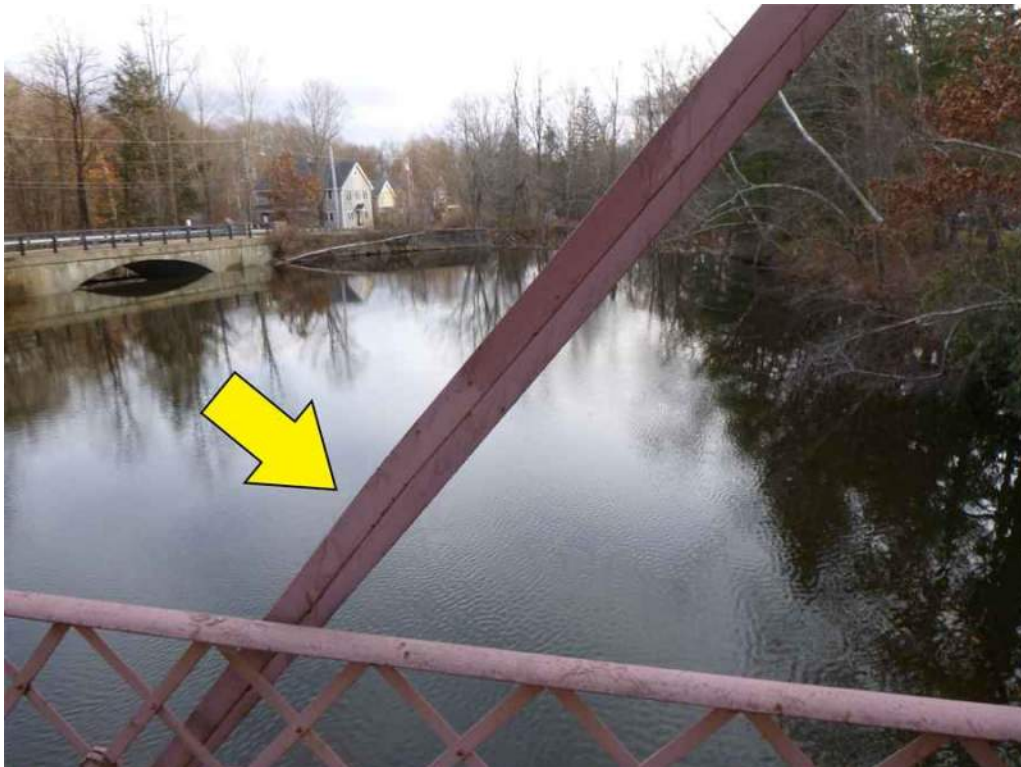
Photo 64: On the south truss, on Diagonal U1 to L2 there is a bend in the web member.
