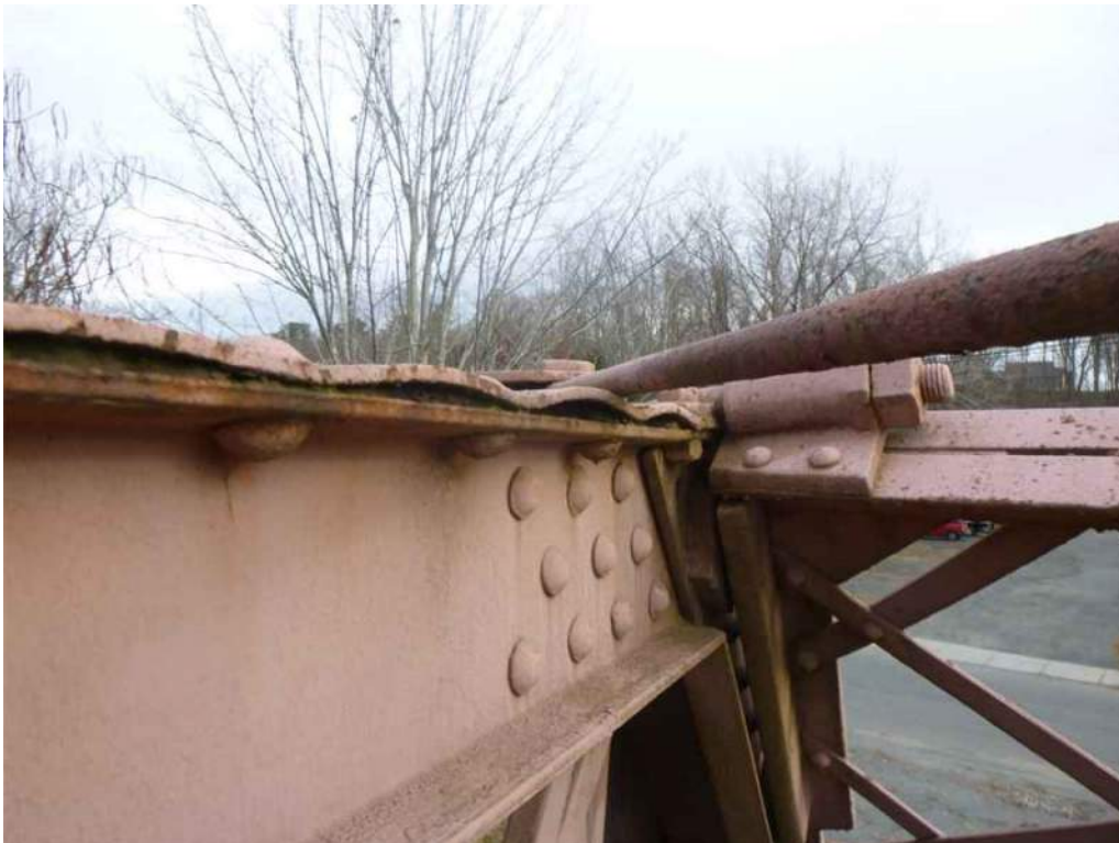
Photo 60: There is up to 2" pack rust between the top plate and the top flange of the c-channel at Panel Point U8.
