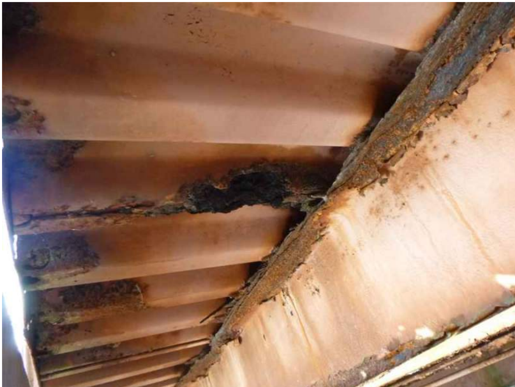
Photo 42: Bay 5, Stringer 4 at Floorbeam 5 has 75% loss of section to top flange of Stringer 4.
