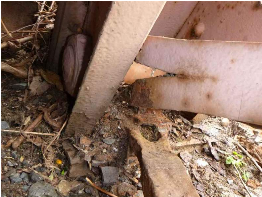
Photo 10: At the east abutment, north truss, Member L9 exhibits up to 10% section loss to the end of the exterior lower chord eye bar.
