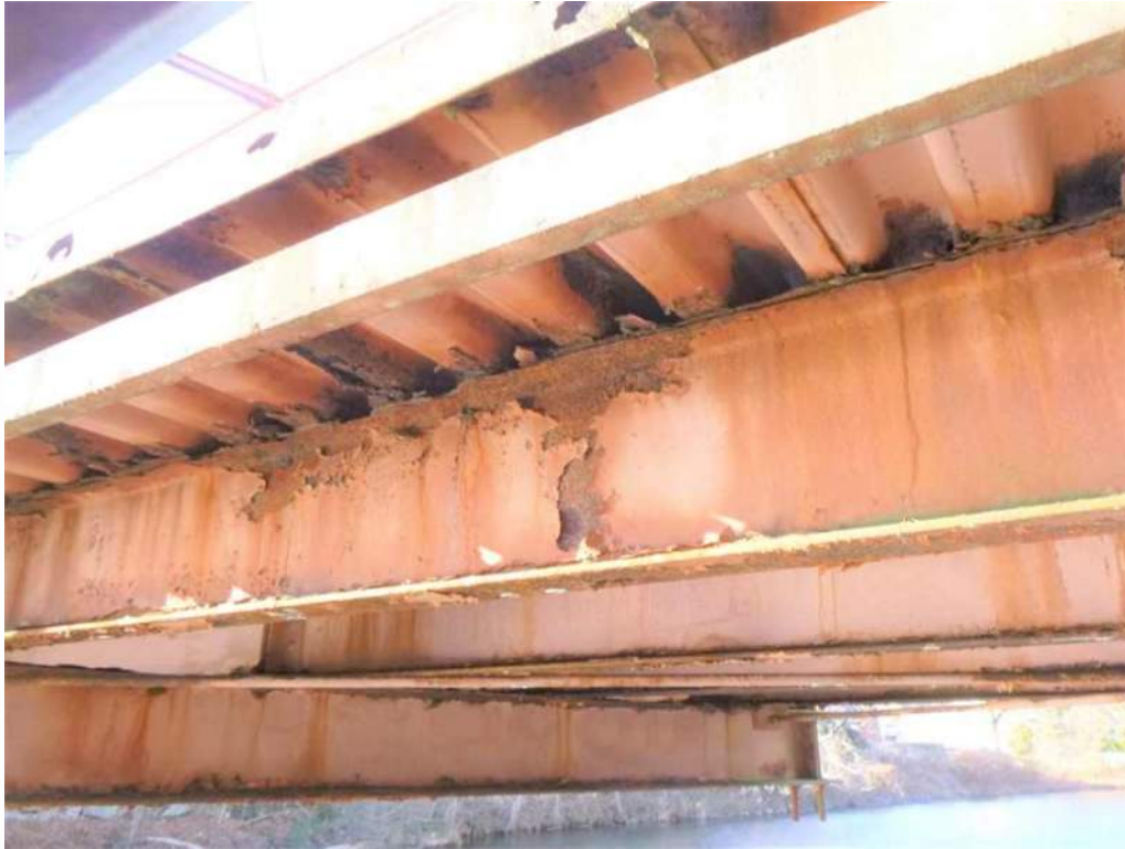
Photo 47: Bay 7, Stringer 1 between Floorbeam 6 and 7 there is 100% loss of section to stringer's top flange.
