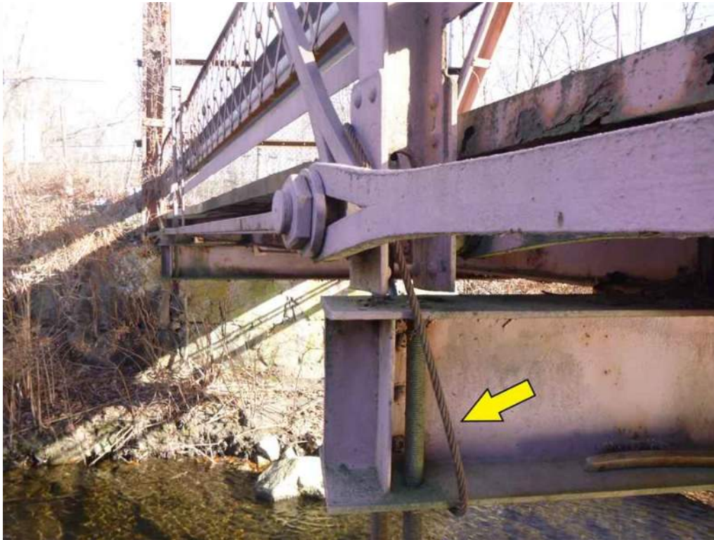
Photo 13: The north U-bolt hanger at Floorbeam 7 has broken at the top of the coupling nuts and has been replaced with a steel cable that connects the floorbeam to the diagonal eye-bar member (Photo 1 of 2).
