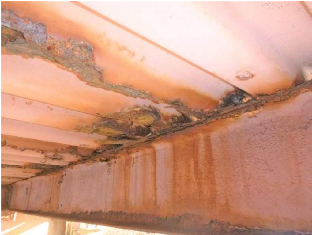
Photo 44: Bay 6, Stringer 1 between Floorbeam 5 and 6 has 75% loss of section to stringer's top flange.
