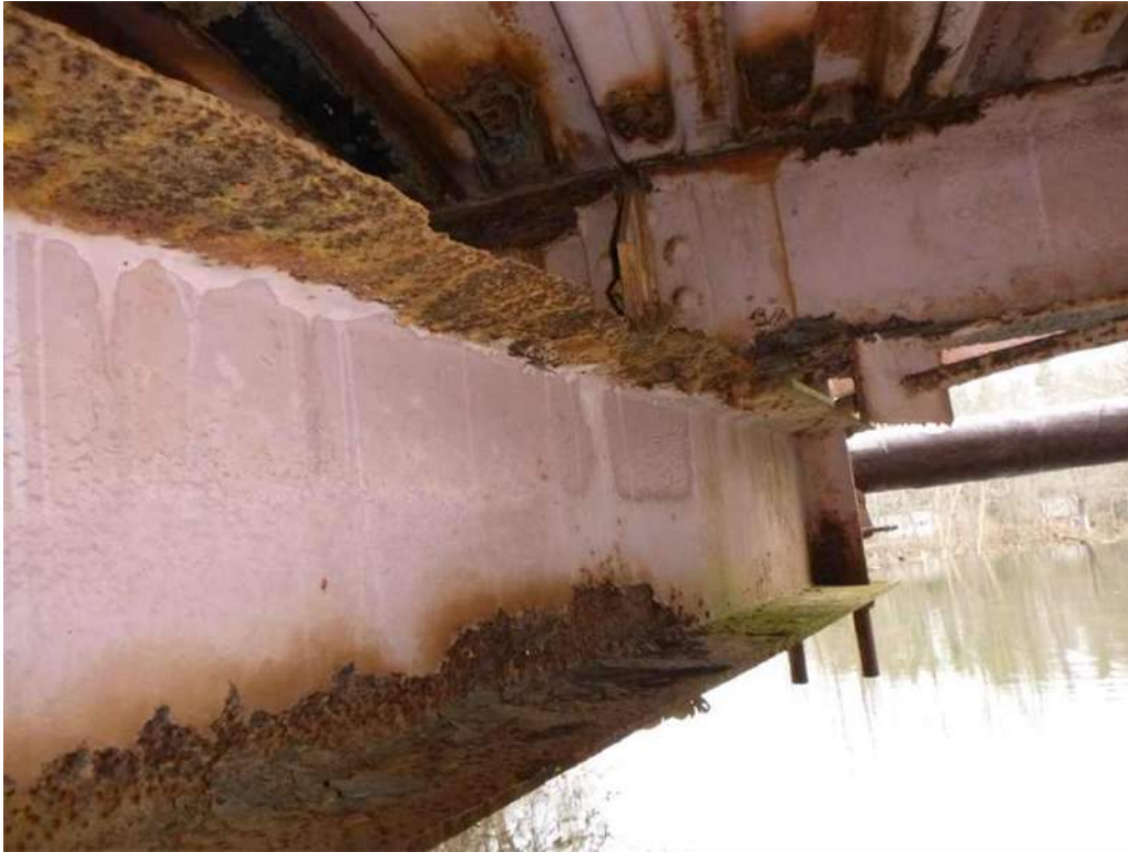
Photo 3: 100% loss of section and knife edging at the top flange of the west face of Floorbeam 7 between Stinger 1 and 2.
