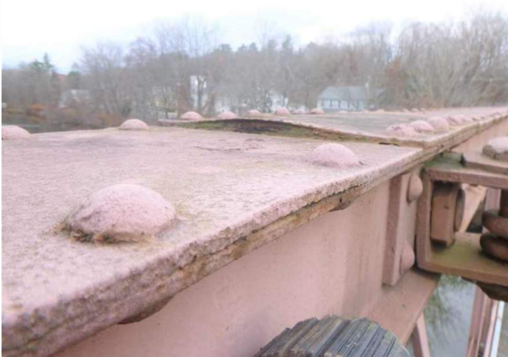
Photo 57: There is up to 2" of pack rust at Panel Point U2.
