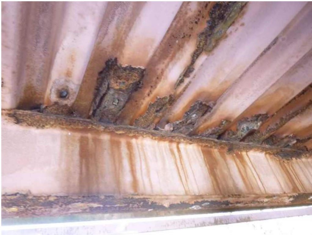
Photo 30: Bay 7, south overhang, multiple 8" wide sections with 100% section loss to corrugated steel deck.
