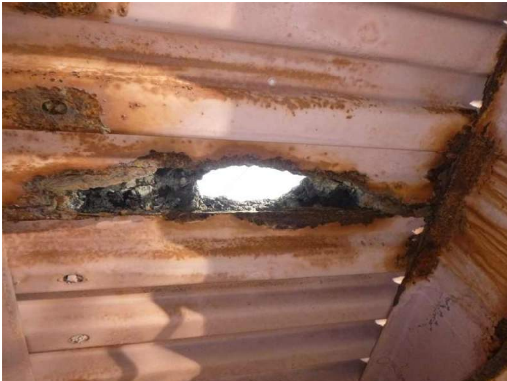
Photo 20: Midspan of Bay 4, 9" wide x 4" long hole with 100% section loss between Stringers 3 and 4.
