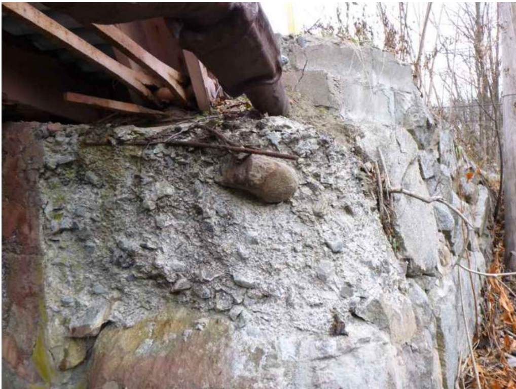
Photo 74: The east abutment has 42" wide x 27" long x 24" deep spall with exposed and corroded rebar at south end of the truss.
