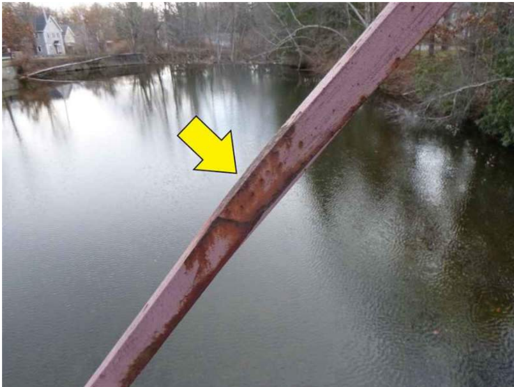
Photo 12: South truss, Diagonal U2 to L3 there is a bend in the web member.
