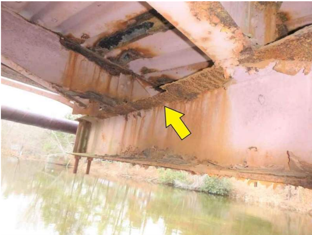
Photo 52: 100% loss of section and knife edging at the top flange of the east face of Floorbeam 7 between Stringers 1 and 2.
