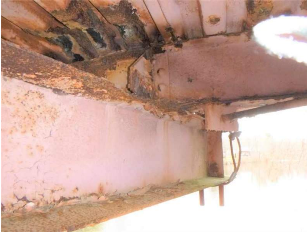
Photo 5: 100% loss of section and knife edging at the top flange of the east face of Floorbeam 7 at Stringer 4.
