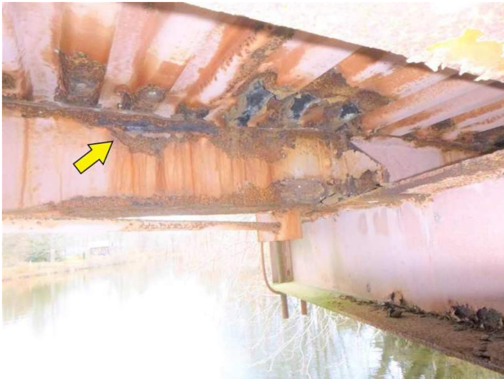
Photo 48: Bay 7, Stringer 4 at Floorbeam 7 there is 100% loss of section to the top flange and the web of Stringer 4.
