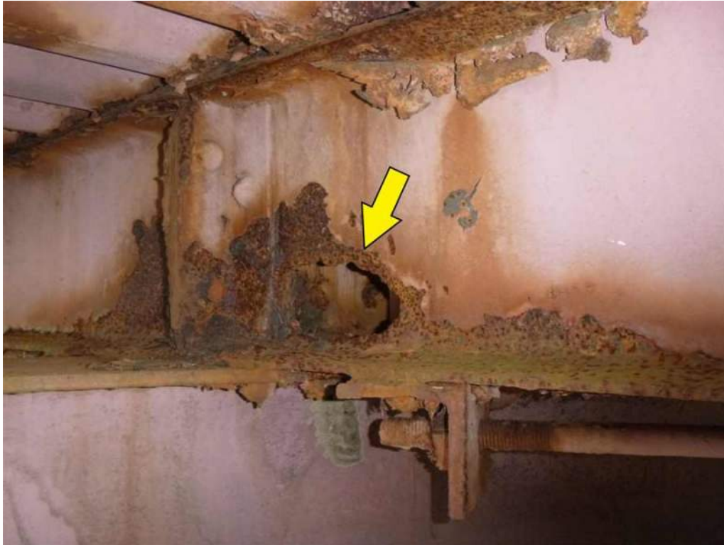
Photo 41: Bay 3, Stringer 4 at Floorbeam 3 has a 6" long by 3" wide hole with 100% loss of section to web.
