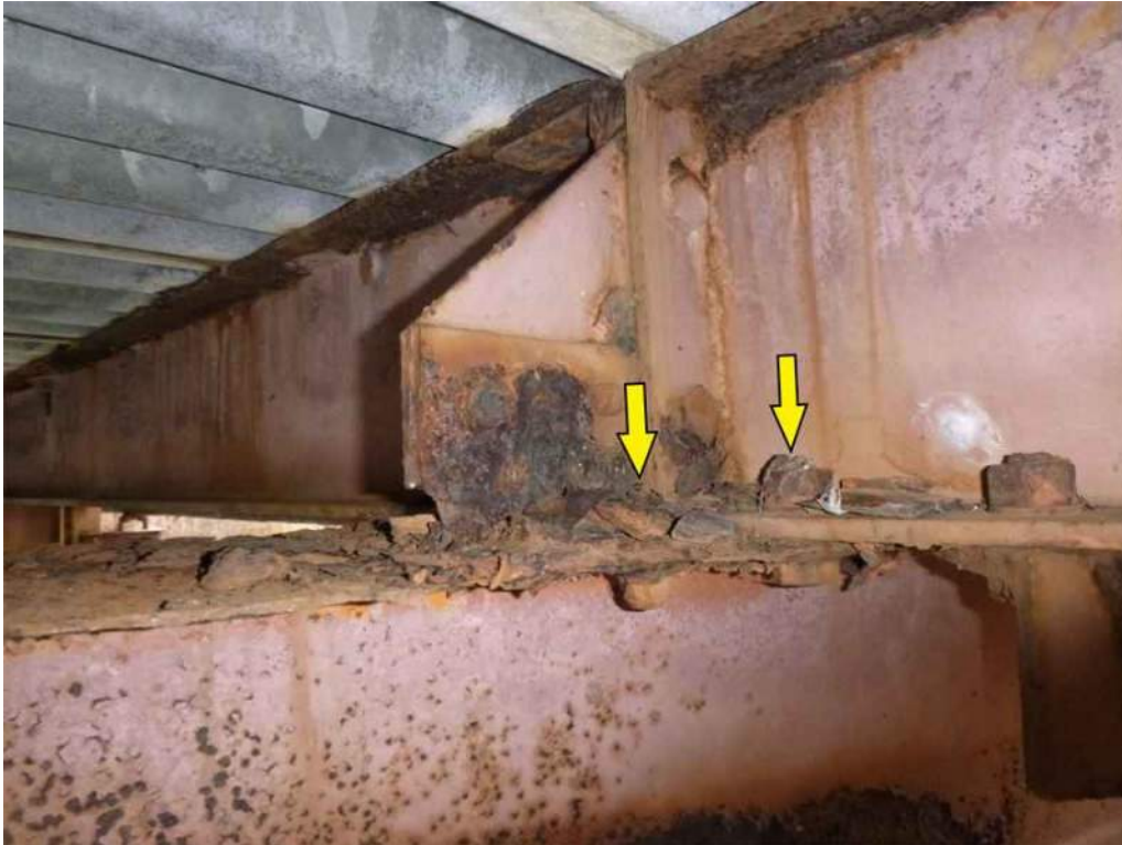
Photo 73: The Stringer 1 bearing stiffener at Floorbeam 2, has up to 100% loss of section to the horizontal rivet heads on top of the floorbeam/stringer connection.
