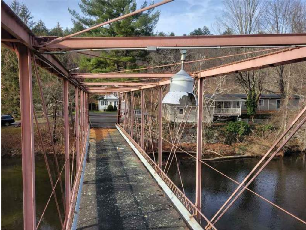
Photo 37: Two lamps on bridge that are attached to top strut. Lamps are broken.
