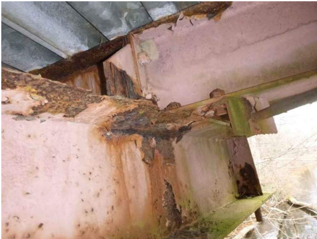
Photo 50: 100% loss of section to the top flange of Floorbeam 1 at Stringer 4.
