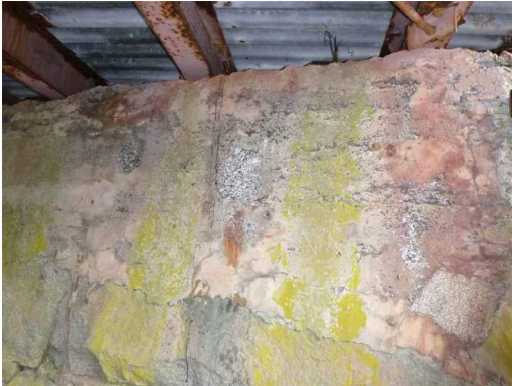
Photo 77: The east abutment between Stringers 1 and 2 has missing mortar and scaling at the top 2 feet of the abutment.
