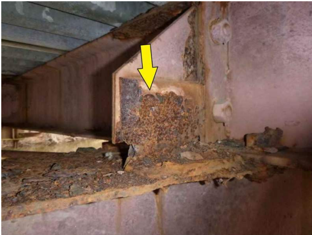
Photo 40: Bay 2, Stringer 1 at Floorbeam 2 has 100% loss of section to bolt head connecting floorbeam to stringer.
