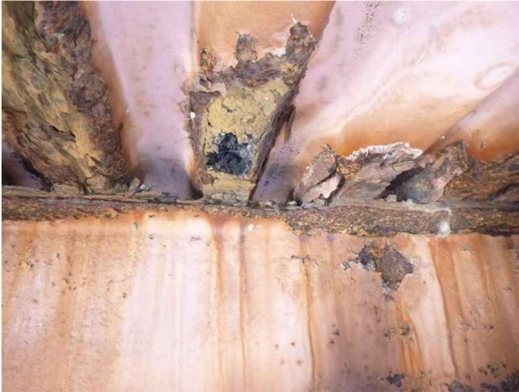
Photo 45: Bay 6, Stringer 4 between Floorbeam 5 and 6 there is 75% loss of section to stringer's top flange, 3' from Floorbeam 5.
