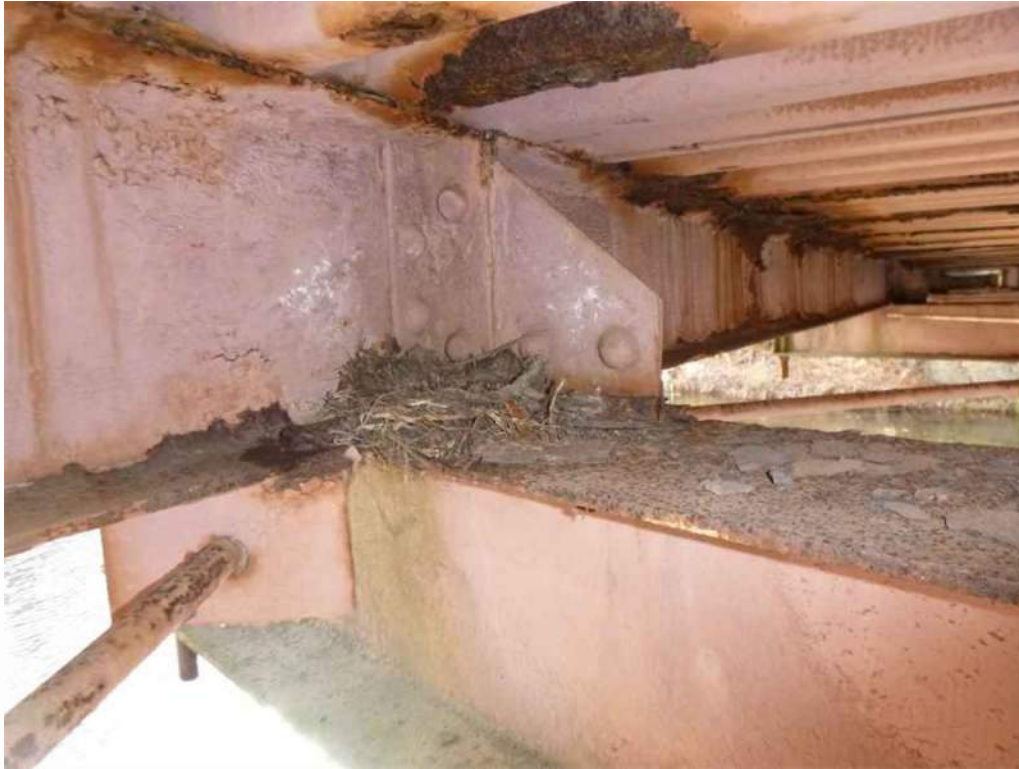
Photo 43: Bay 6, Stringer 1 at Floorbeam 5 there is a bird's nest.
