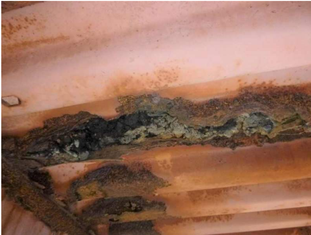
Photo 21: Bay 4, 2'-0" wide hole, 100% section loss to bottom of corrugated steel deck between Stringers 1 and 2.
