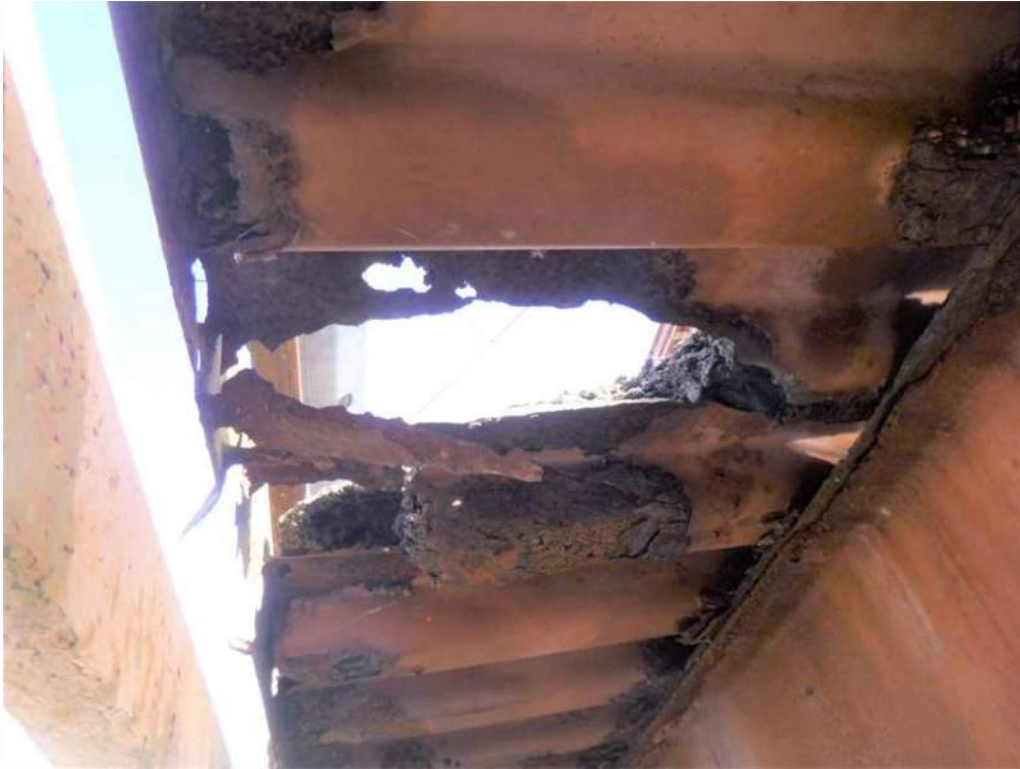
Photo 25: Bay 6, north overhang, 12" wide x 6" long hole with 100% section loss to corrugated steel deck.
