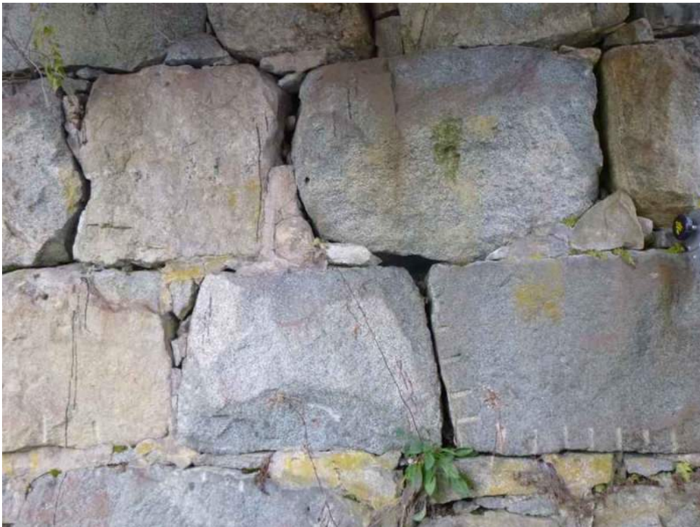
Photo 78: The west abutment is missing mortar and has failed pointing. There is typical cracked pointing and vegetation growth in joints (Photo 1 of 2).
