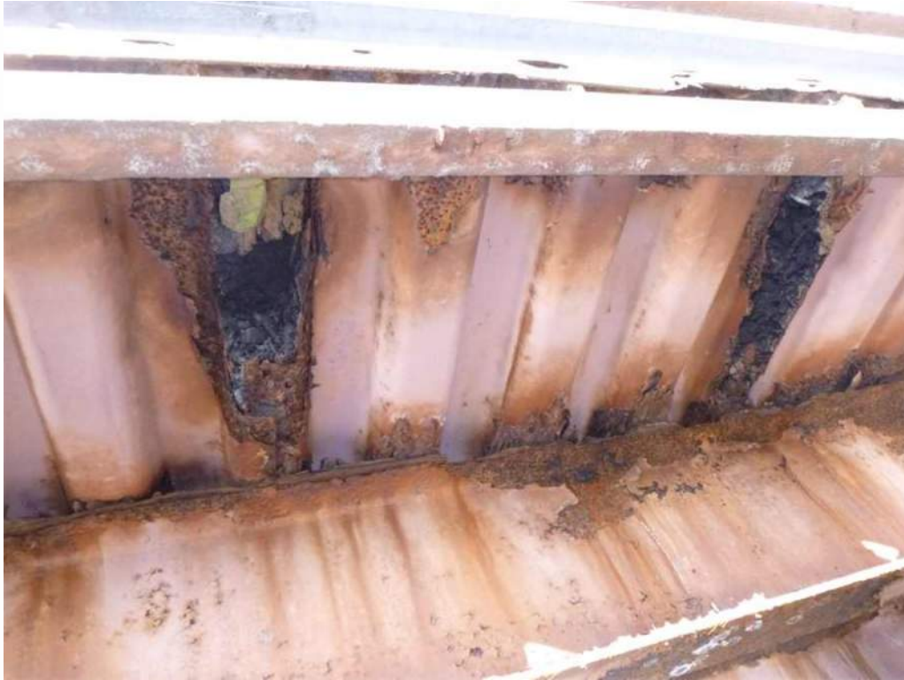
Photo 29: Bay 7, north overhang, multiple 12" wide sections with 100% section loss to corrugated steel deck.
