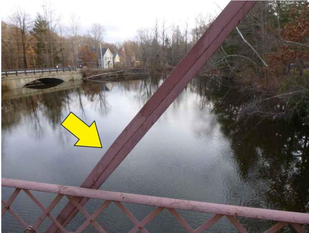
Photo 11: On the south truss, on Diagonal U1 to L2 there is a bend in the web member.
