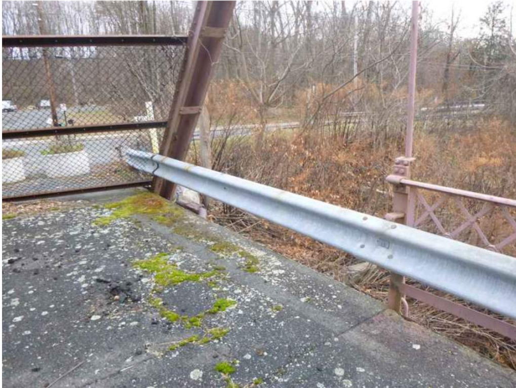
Photo 35: Both horizontal members and cross-braces are missing for Bay 1, on the south railing.
