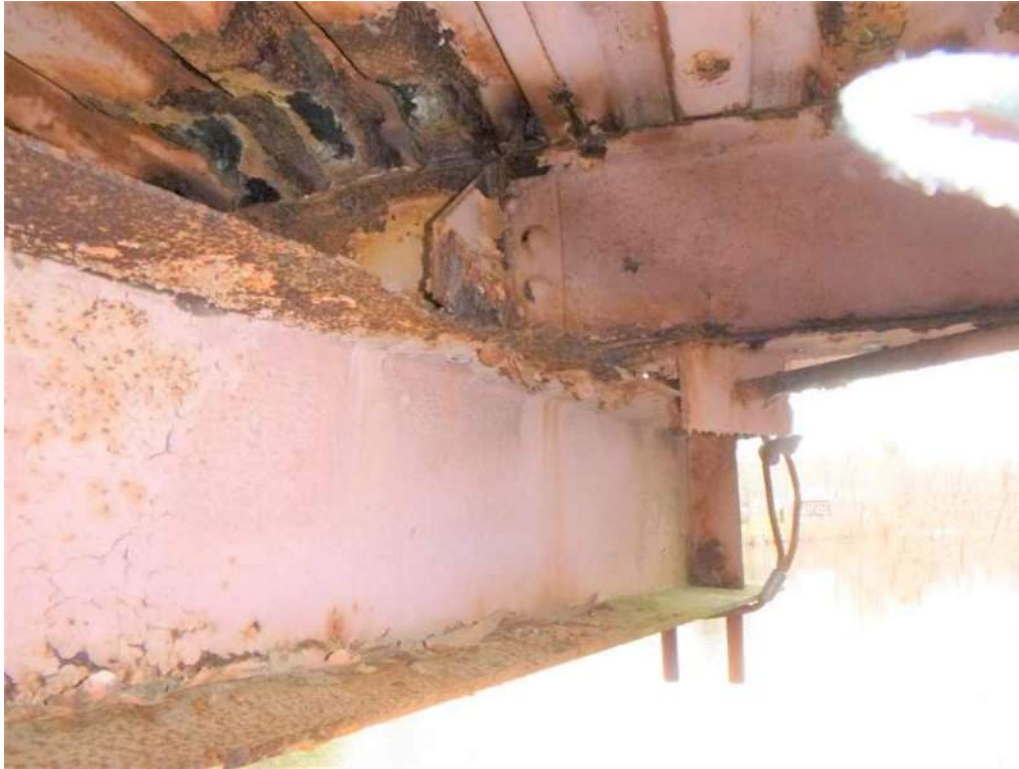
Photo 53: 100% loss of section and knife edging at the top flange of the east face of Floorbeam 7 at Stringer 4.
