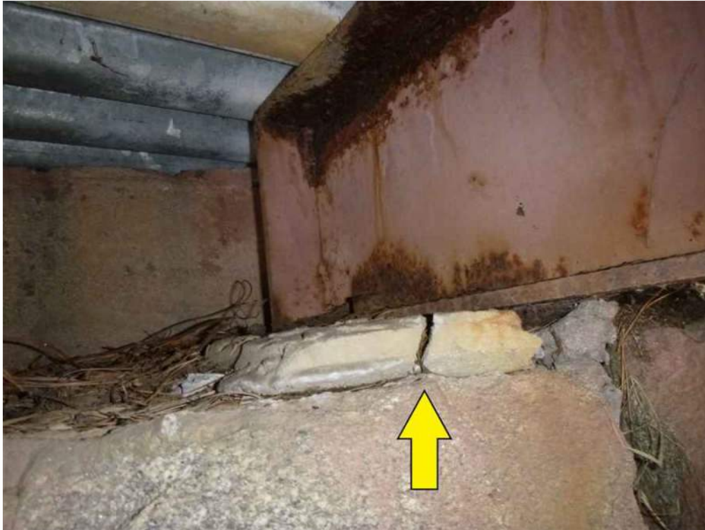
Photo 71: Under Stringer 2 the grout has completely failed.
