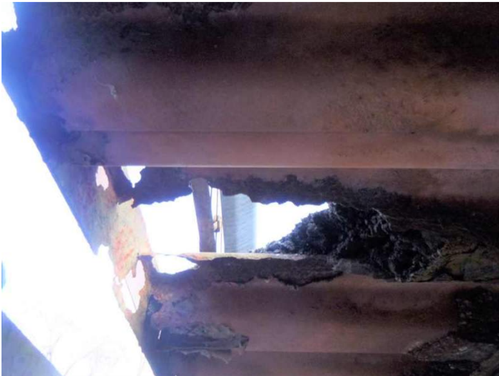
Photo 26: Bay 6, north overhang, 9" wide x 4" long hole with 100% section loss to corrugated steel deck.
