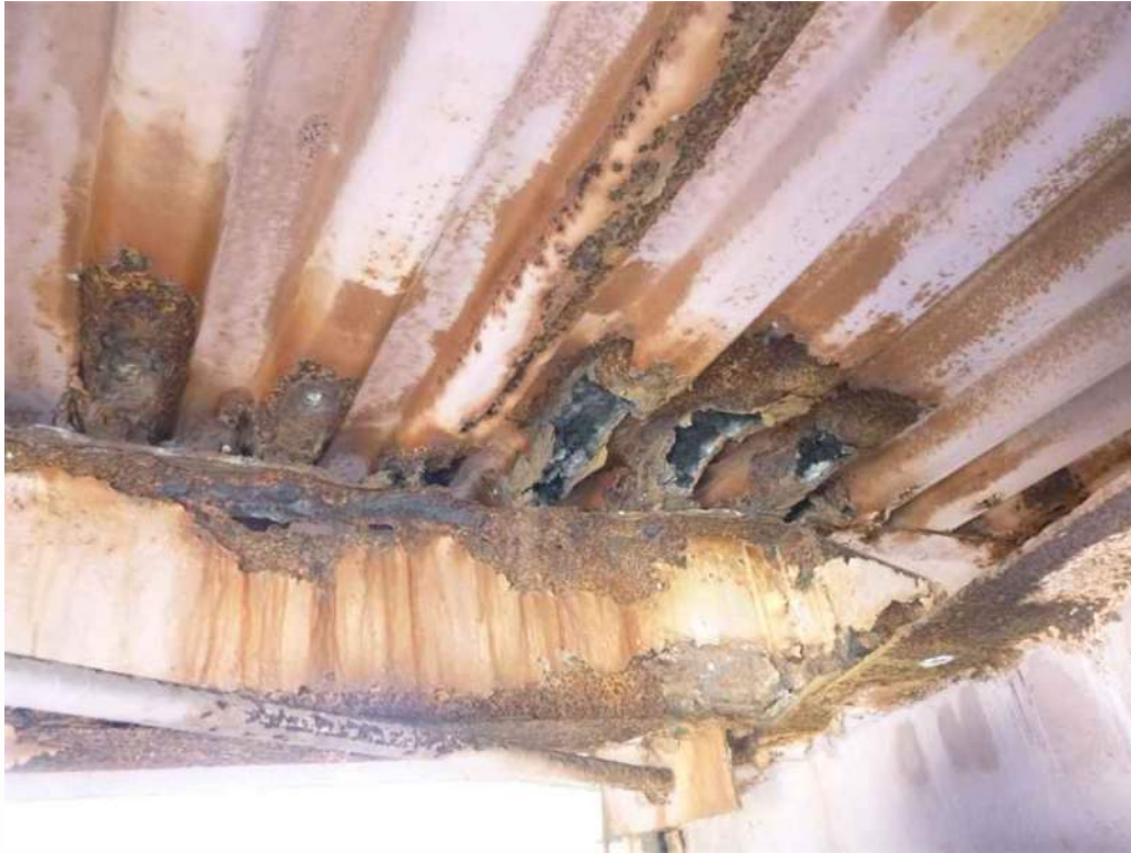
Photo 31: Bay 7, multiple 12" wide sections with 100% section loss to corrugated steel deck (1 of 2).
