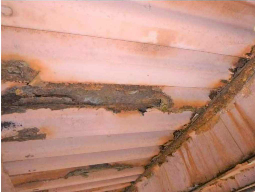
Photo 19: Bay 4, 2'-6" wide, 100% section loss to bottom of corrugated steel deck between Stringers 3 and 4.
