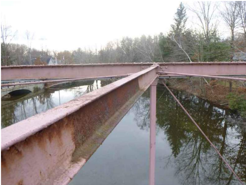
Photo 66: Strut Member U4 north to U4 south exhibits paint failure and corrosion at midspan.
