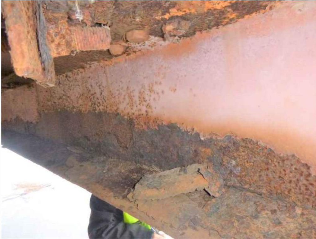
Photo 49: 1/8" loss of section to the web along the entire length of Floorbeam 1.
