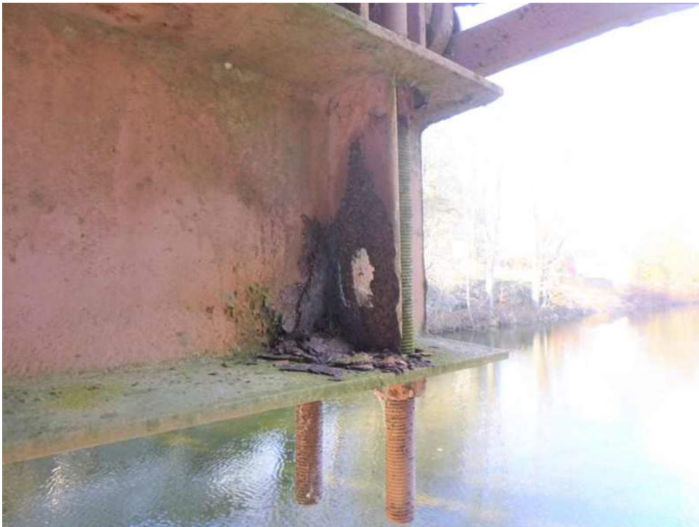
Photo 8: North end of Floorbeam 8 has a 3" long by 2" wide corrosion hole in the stiffener. Laminar corrosion has initiated on the lower half of the web adjacent to the stiffener.
