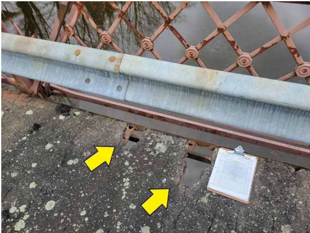
Photo 18: On the north side of the deck, east of Floorbeam 6 there are multiple holes.
