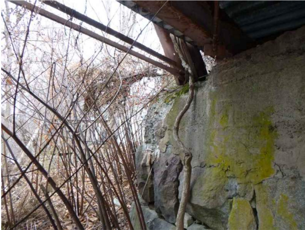
Photo 75: At the east abutment by the north end of truss there is vegetation growth.
