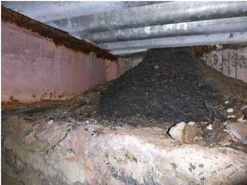
Photo 70: By Stringer 3 on the south side the abutment is completely covered with asphalt.
