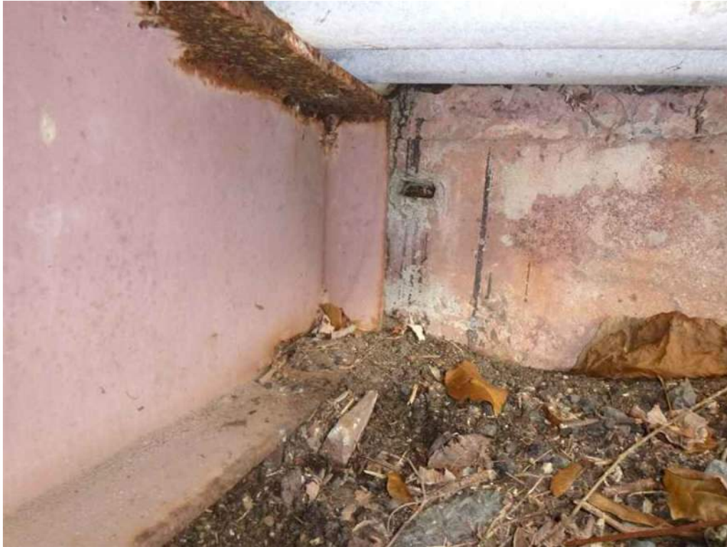
Photo 69: Stringer 1 bearing on east abutment has heavy debris buildup on bearing.
