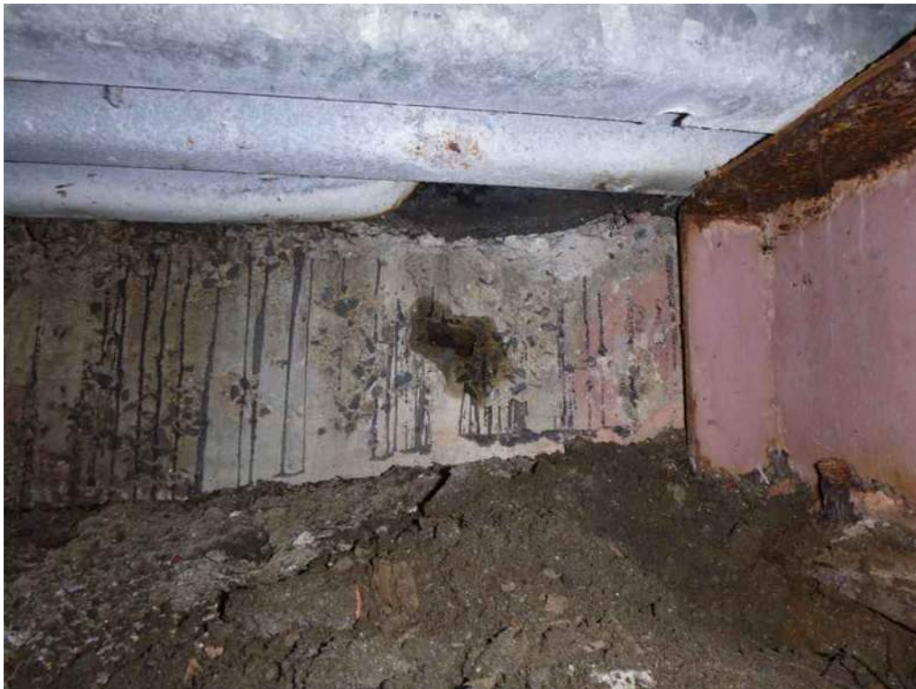
Photo 76: Between Stringers 2 and 3 at the east backwall there is a 3' wide by 1" high by 2" deep spall. There is scaling on the backwall.
