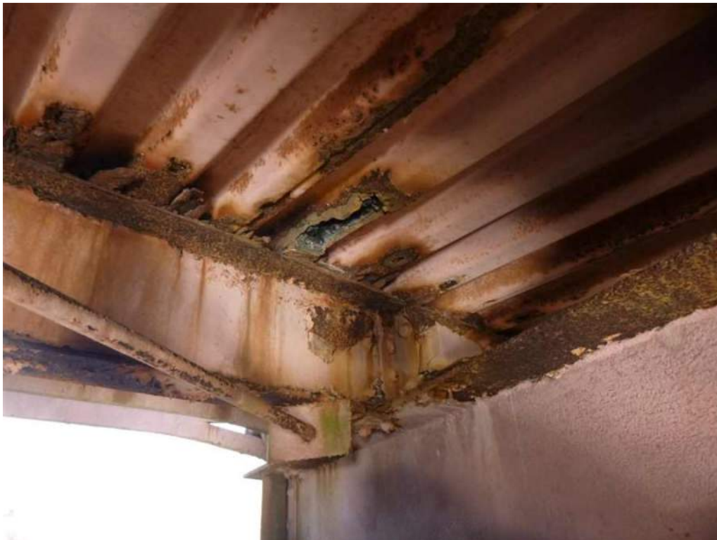
Photo 28: Bay 6, 10" wide hole, 100% section loss to corrugated steel deck between Stringers 3 and 4.
