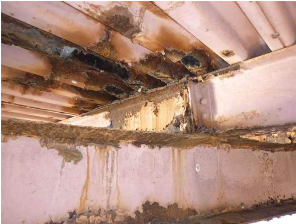
Photo 32: Bay 7, multiple 12" wide sections with 100% section loss to corrugated steel deck (2 of 2).
