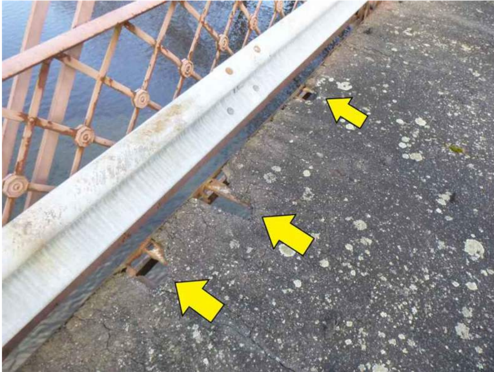
Photo 17: On the north side of the deck, east of Floorbeam 5 there are multiple holes.
