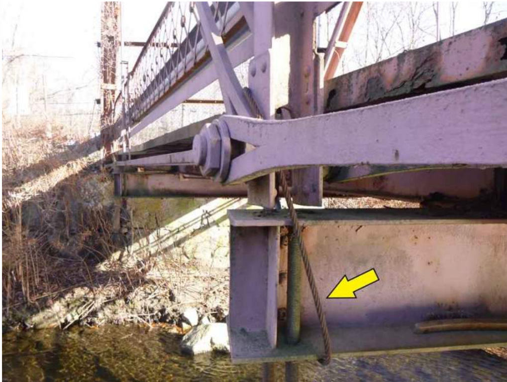
Photo 67: The north U-bolt hanger at Floorbeam 7 has broken at the top of the coupling nuts and has been replaced with a steel cable that connects the floorbeam to the diagonal eyebar member (Photo 1 of 2).
