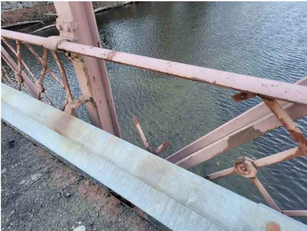
Photo 34: On the north truss, at Panel Point 6, the cross bracing is missing.
