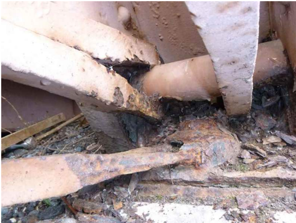
Photo 62: South truss at L9 has 1/8" section loss with active surface corrosion to the end of the interior lower chord eye bar.
