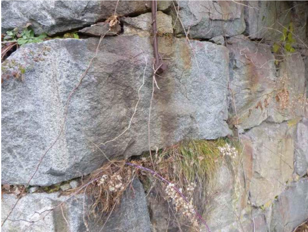
Photo 79: The west abutment is missing mortar and has failed pointing. There is typical cracked pointing and vegetation growth in joints (Photo 2 of 2).
