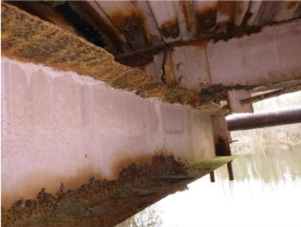
Photo 51: 100% loss of section and knife edging at the top flange of the west face of Floorbeam 7 between Stringer 1 and 2.
