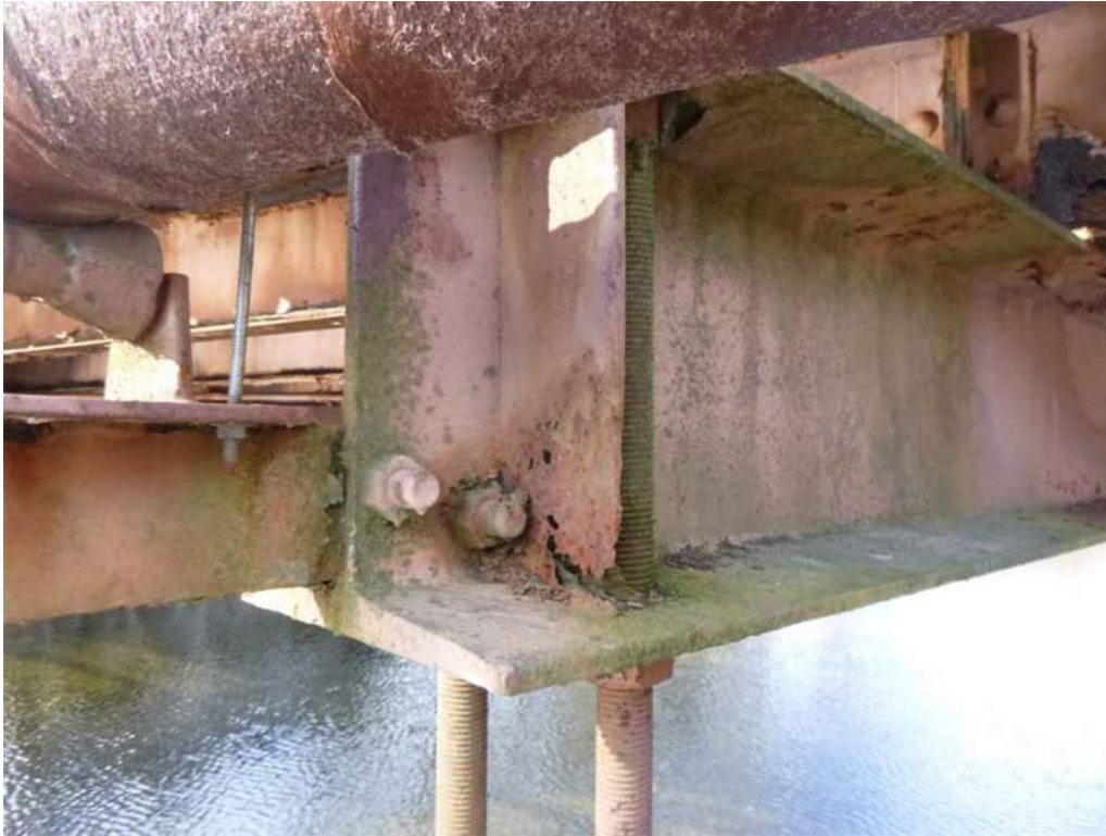
Photo 7: Floorbeam 8, on the south end has up to 50% section loss to the stiffener.
