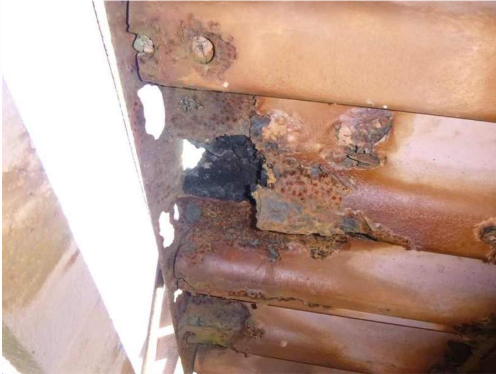
Photo 27: Bay 6, north overhang, 7" wide x 5" long hole with 100% section loss to corrugated steel deck.
