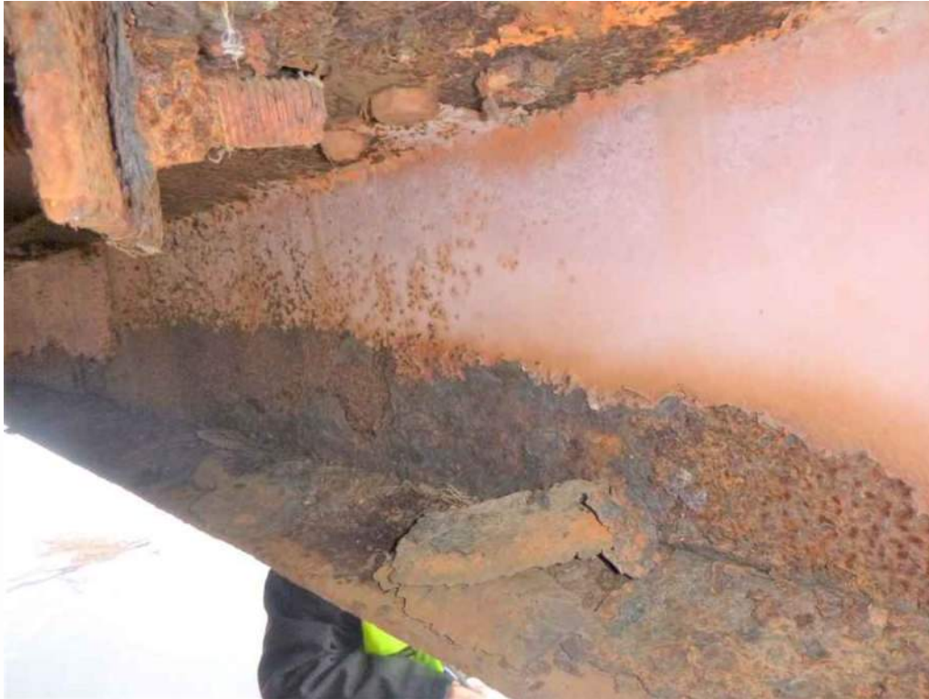
Photo 1: 1/8" loss of section to the web along the entire length of the Floorbeam 1.
