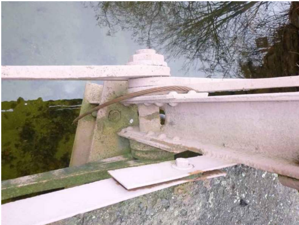
Photo 68: The north U-bolt hanger at Floorbeam 7 has broken at the top of the coupling nuts and has been replaced with a steel cable that connects the floorbeam to the diagonal eyebar member (Photo 2 of 2).
