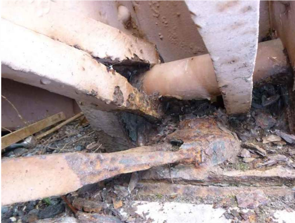
Photo 9: South truss at L9 has 1/8" section loss with active surface corrosion to the end of the interior lower chord eye bar.
