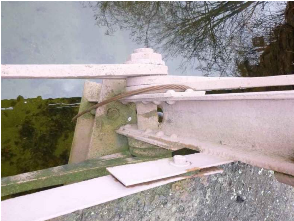
Photo 14: The north U-bolt hanger at Floorbeam 7 has broken at the top of the coupling nuts and has been replaced with a steel cable that connects the floorbeam to the diagonal eye-bar member (Photo 2 of 2).
