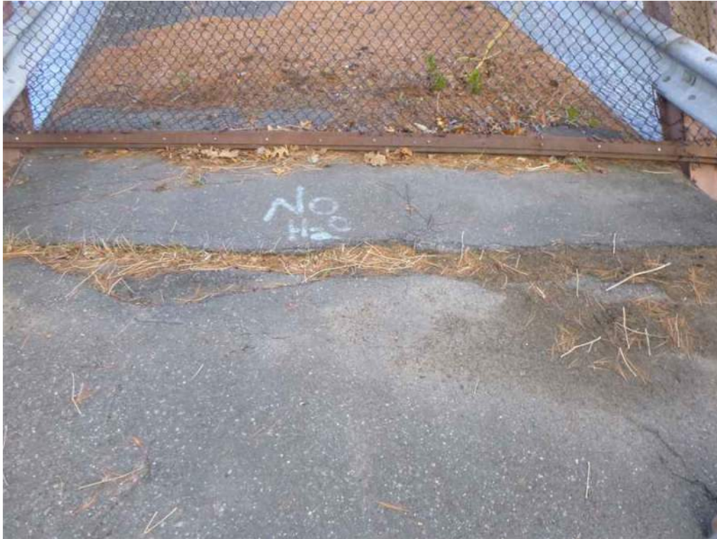
Photo 11: Asphalt patch at the west end of the bridge (no joint found).
