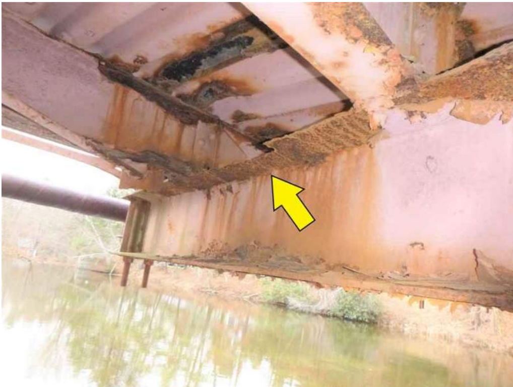
Photo 4: 100% loss of section and knife edging at the top flange of the east face of Floorbeam 7 between Stringers 1 and 2.
