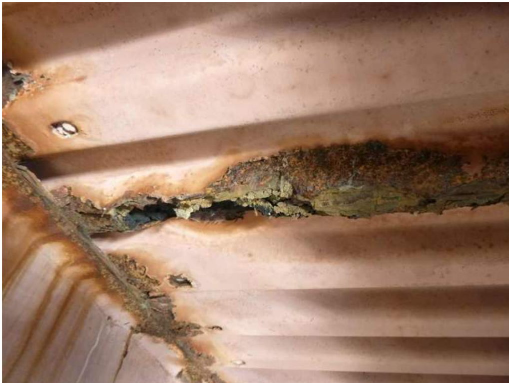
Photo 22: Bay 5, 2'-0" wide hole, 100% section loss to bottom of corrugated steel deck between Stringers 3 and 4.
