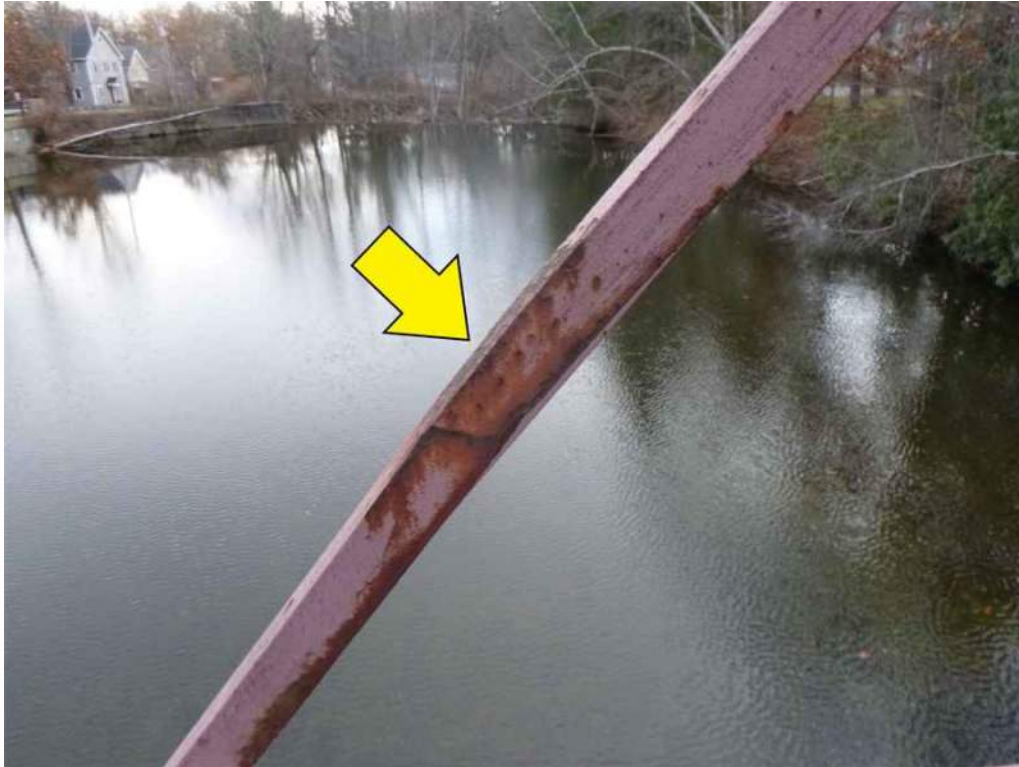
Photo 65: South truss, Diagonal U2 to L3 there is a bend in the web member.
