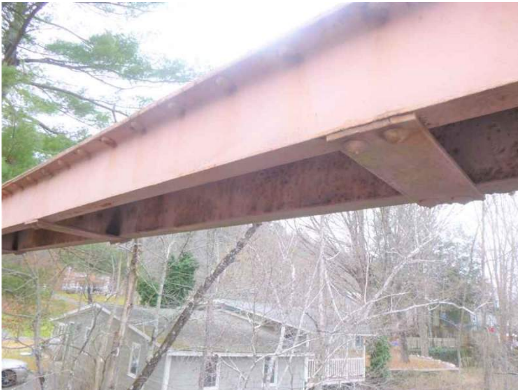
Photo 58: The inside of both c-channels on member U2-U3 have minor to moderate areas of corrosion.
