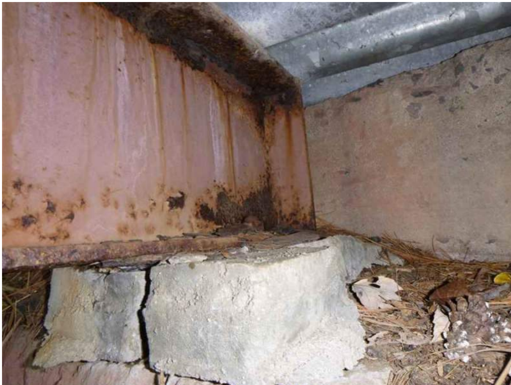
Photo 72: The grout under Stringer 4 at the west abutment is cracked, but the anchor bolt is in good condition.
