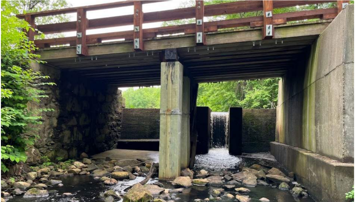
Photo 1: View of the bridge along Winnetuxet Road over the Winnetuxet River in Plympton. Facing northeast.
