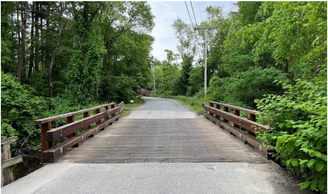
Photo 2: View of the bridge deck and guardrails along Winnetuxet Road. Guardrails appeared to be too open to be suitable for bat use. Facing south.
