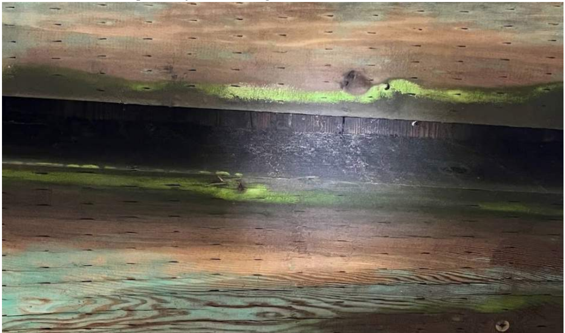
Photo 4: View of the space between wooden beams along the bridge deck. Some debris was observed, which may or may not have been guano, on the side of a wooden beam, but surveyors could not get close enough to accurately decide. Facing south.
