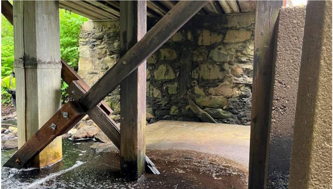
Photo 3: View of the underside of the bridge along Winnetuxet Road in Plympton. No bats were observed in the spaces between the walls, cracks in concrete, spaces between the wooden beams, or expansion joints. Facing north.
