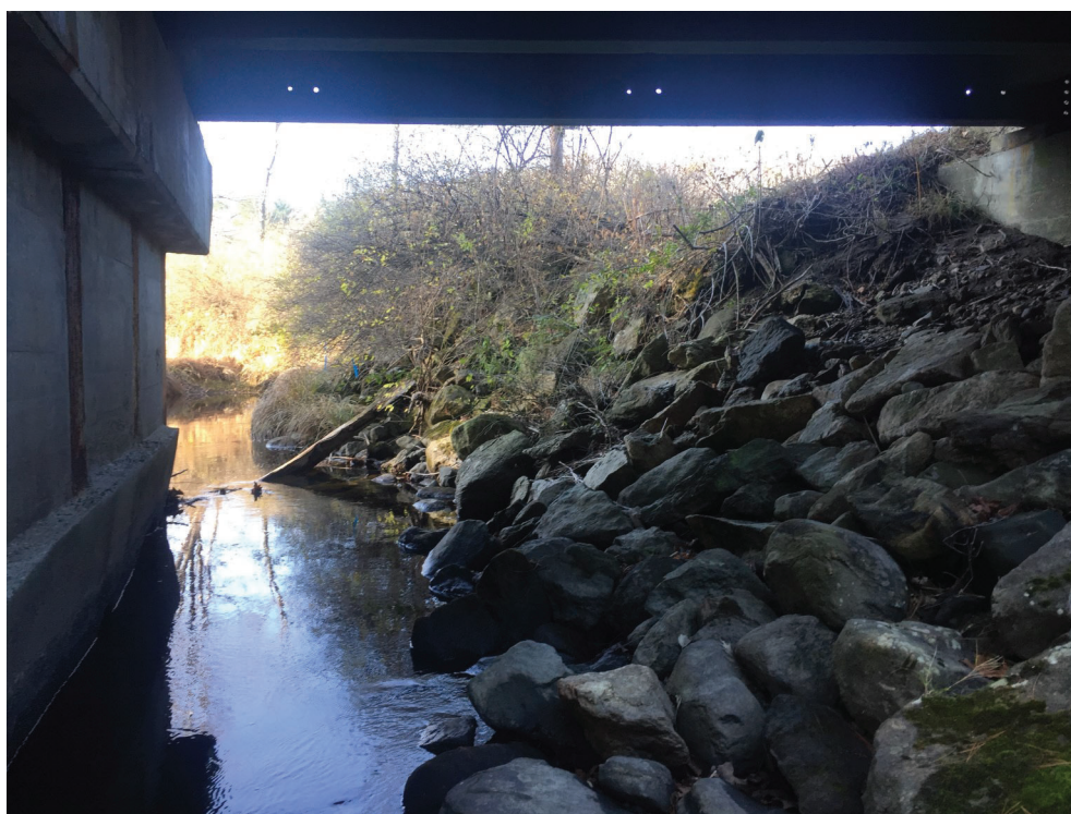
View of the armored Stream Bank adjacent to the northerly bridge abutment—facing west.
