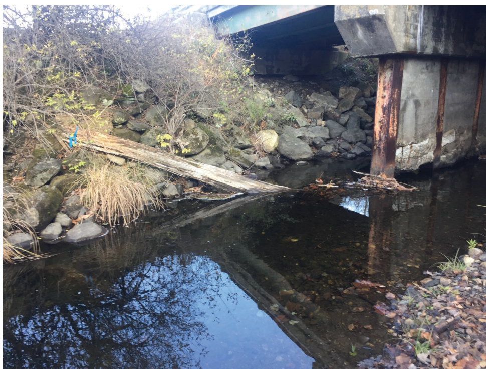
View of the undercut northerly pier—facing northeast.
