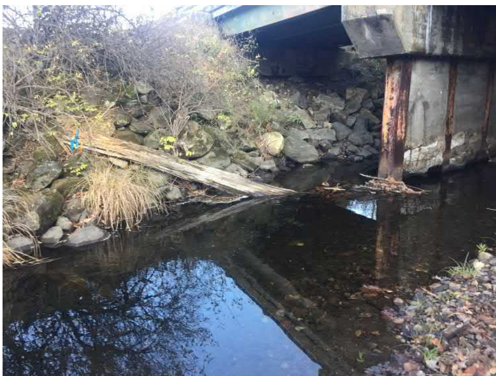
View of the undercut northerly pier—facing northeast.
