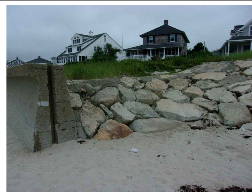
EXISTING REVETMENT AT STA. 29+50 TO BE REMOVED & RECONSTRUCTED
