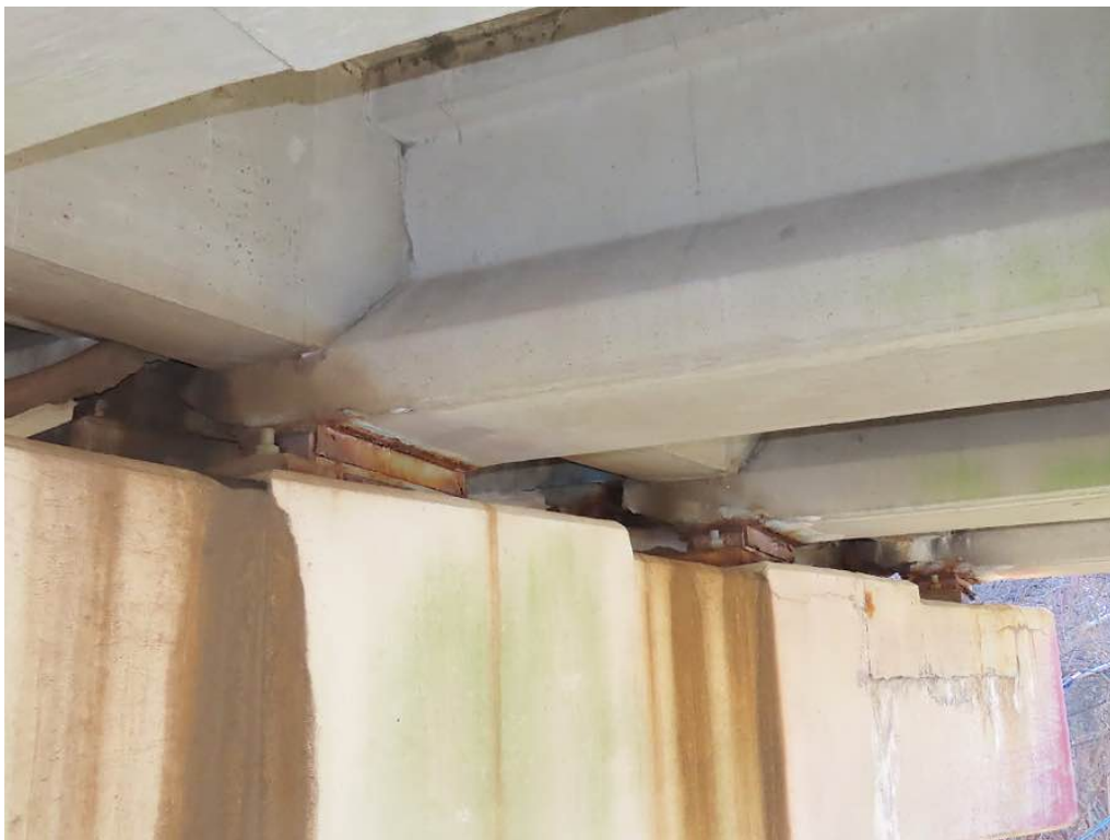
Photo 32: Close up of previous photo 30 - South end of pier 2 cap with horizontal cracking at previous repair location above column 4.
