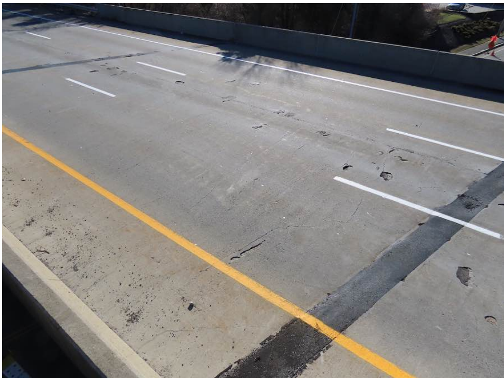
Photo 5: Overview of span 2 concrete deck/wearing surface with transverse cracks and numerous partial filled potholes looking southeast. On the right, pier 1 plug joint.
