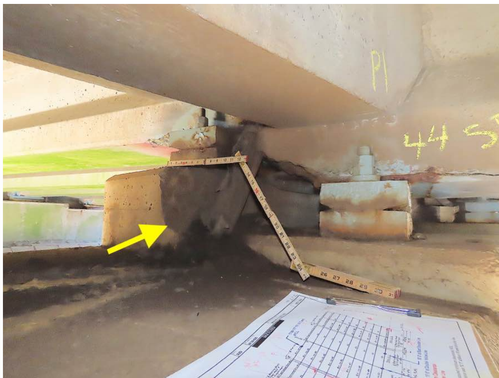
Photo 19: Close up of previous photo 17 - Beam ends 34 and 44 south face at pier 1. Beam 44 with end spall with exposed rebar and delam in front of bearing - Typical. Beam 34 pedestal with SE corner spall (Y).
