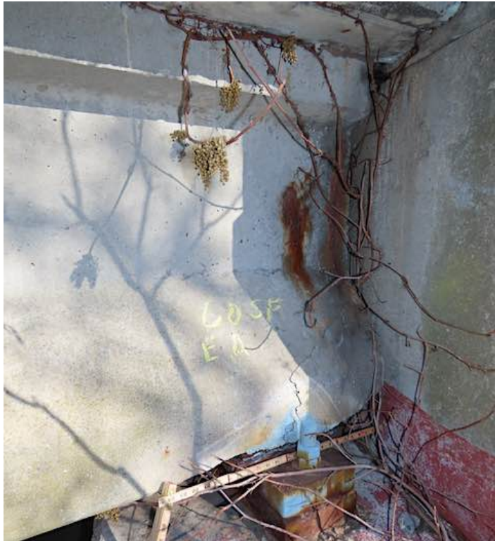
Photo 22: Fascia beam 60, north face at the east abutment with end spall before and after the bearing.
