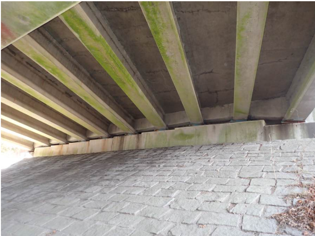
Photo 14: Span 1 looking west, typical condition of algae staining along the beams.
