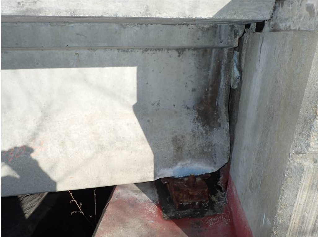
Photo 13: Beam 30 East Abutment, spalling past bearing.
