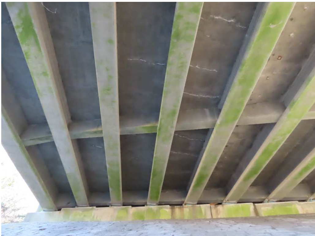
Photo 10: General underside of span 3 looking east, bays 1 through 6 (L to R). Bays with transverse cracks and efflo.
