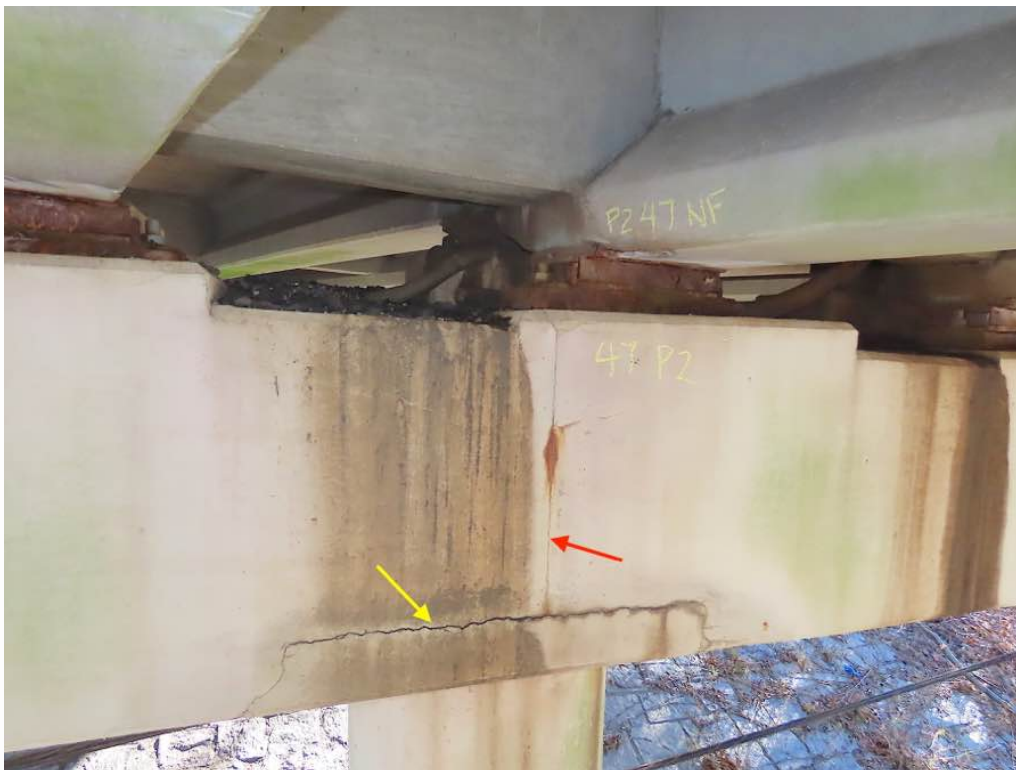
Photo 31: Close up of previous photo - Pier 2 cap with a vertical crack (R) and horizontal crack (Y) at previous repair location above column 3. Heavy debris on top of cap.
