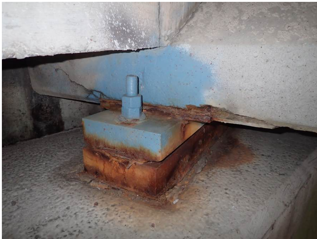
Photo 12: Beam 4 West Abutment, typical condition of horizontal cracking/delamination/spall at the top of the embedded steel bearing plate.
