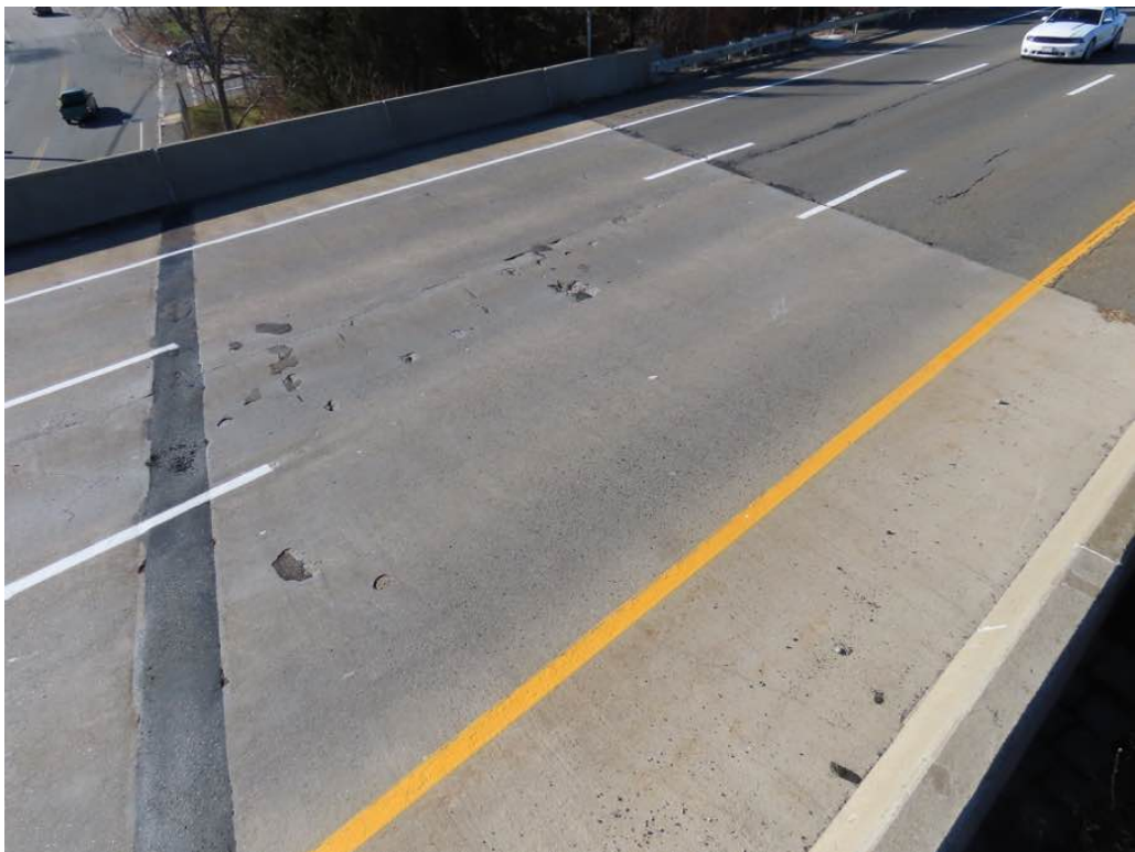
Photo 4: Overview of span 1 concrete wearing surface looking south. On the left, pier 1 plug joint.
