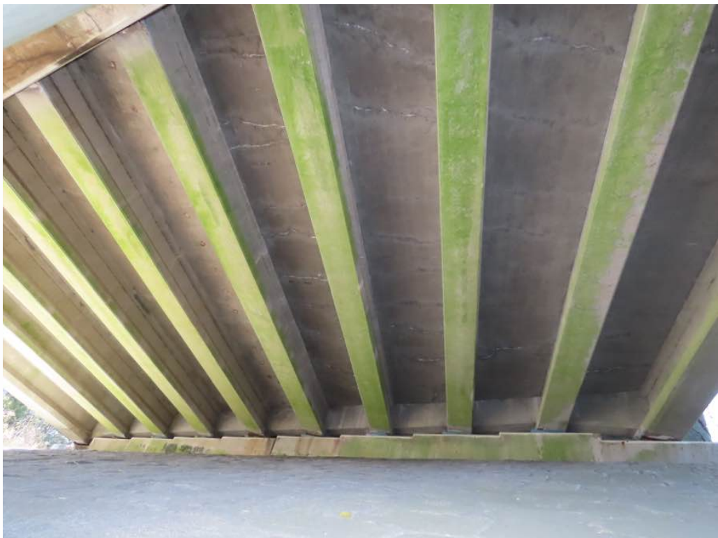
Photo 7: General underside of span 1 looking west, bays 9 through 1 (L to R). Bays with transverse cracks and efflo. Overview of west breastwall.
