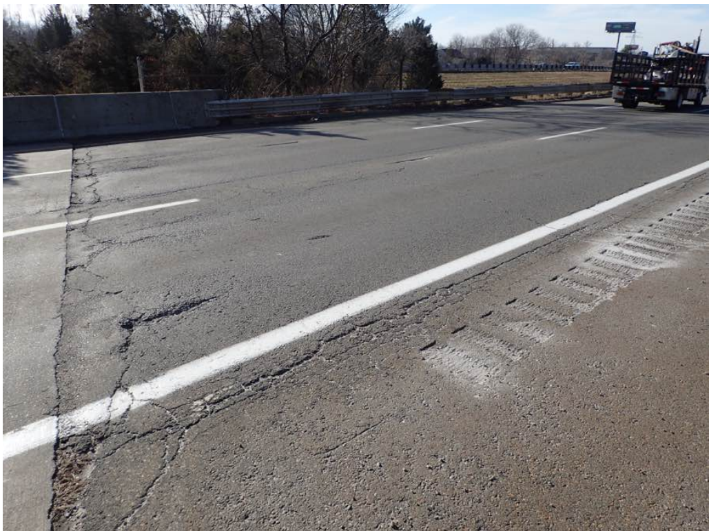
Photo 10: West Approach looking southwest, typical condition with wheel rutting and cracking.
