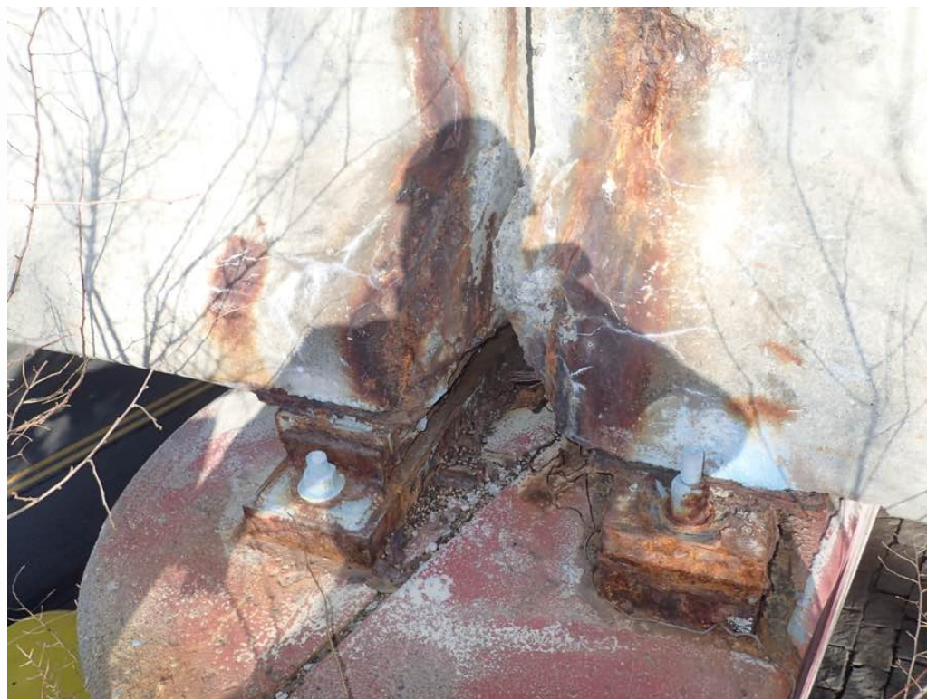
Photo 17: Beam 30 Pier 2 south face, spalling with exposed rebar.
