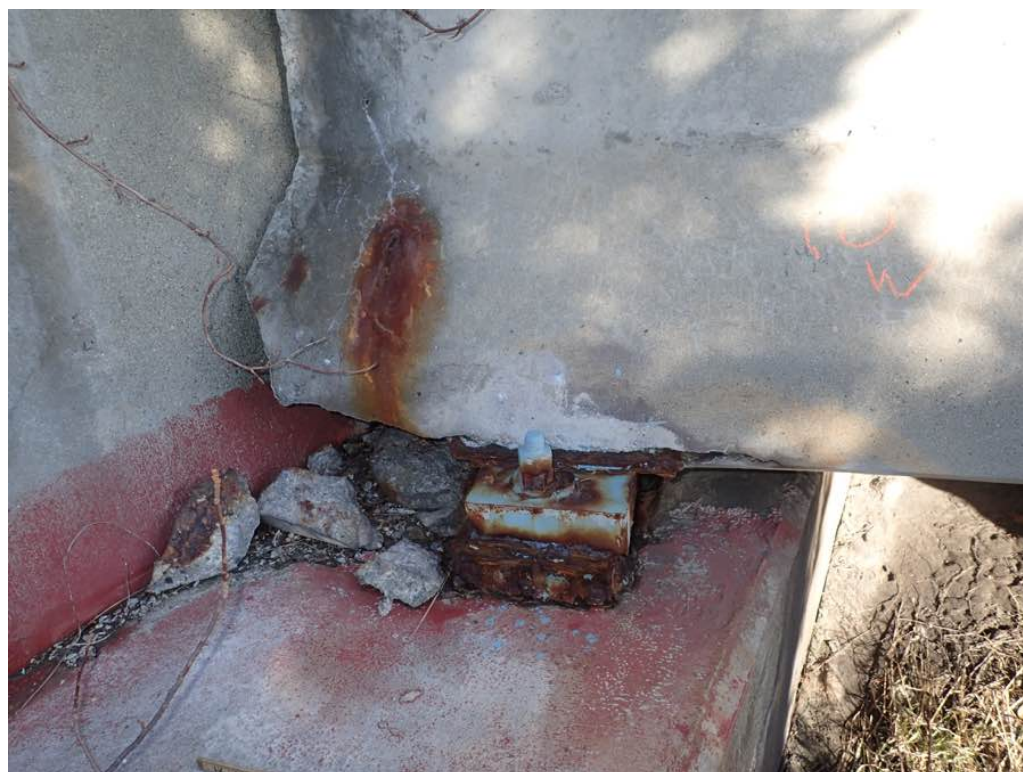
Photo 18: Beam 10 West Abutment, typical condition of bearing corrosion.
