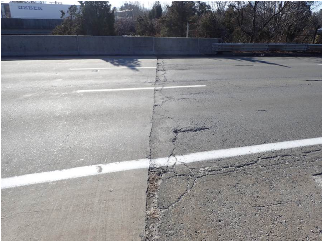
Photo 8: West Abutment looking south, approach pavement breaking up.
