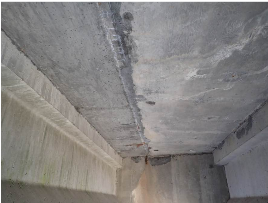
Photo 3: Span 2 Bay 5 looking east, typical condition of efflorescence along the construction joint.
