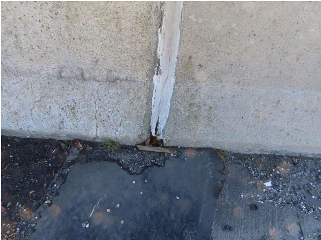
Photo 14: Pier 1 joint at south parapet with hole at the joint. Pier 2 joint at south parapet is similar.
