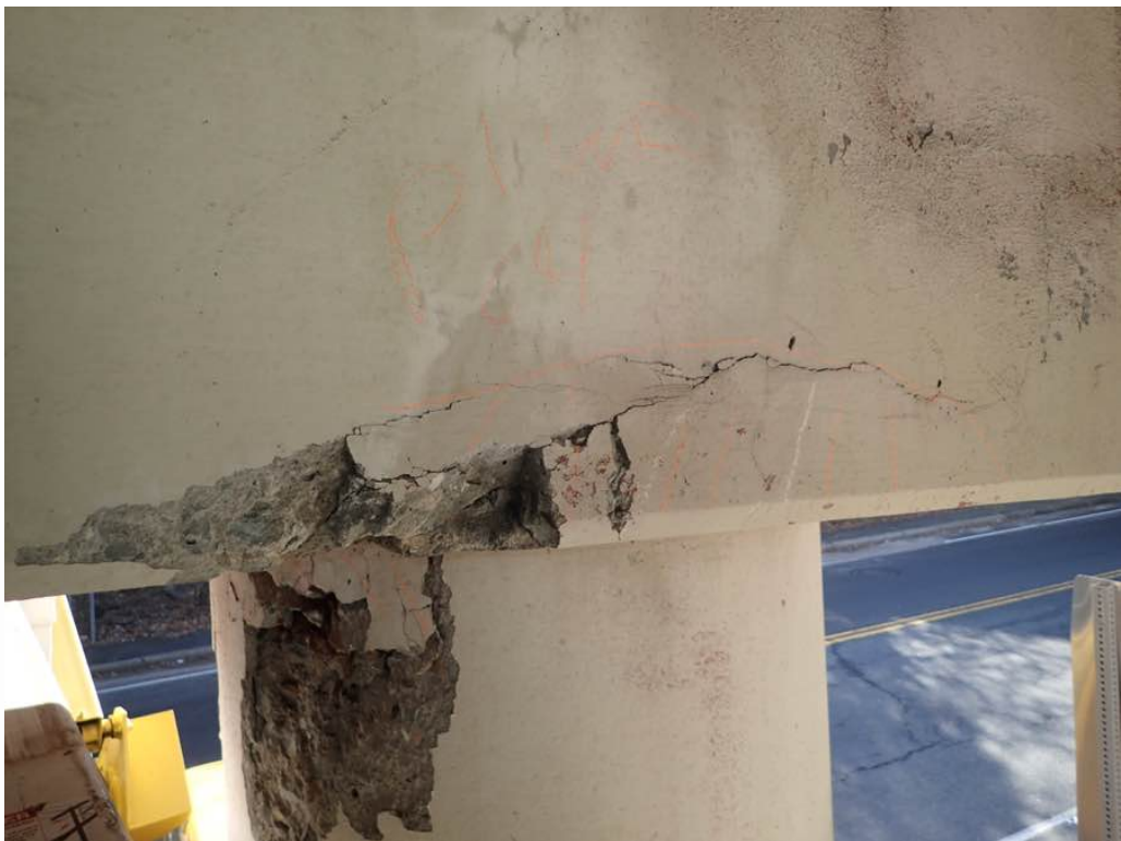
Photo 21: Pier 1 west face above Column 4, spall/delamination.
