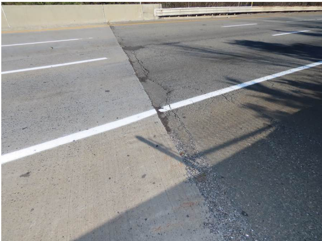
Photo 15: Overview of east approach pavement along the span 3 concrete wearing surface looking north. Approach pavement with curb to curb cracking, settlement, and settled patches.
