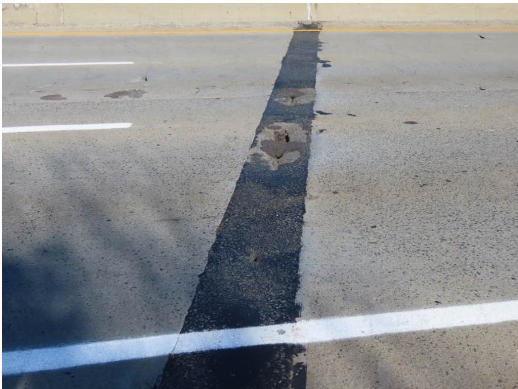
Photo 13: Overview of pier 2 joint looking north. Settled holes in right and center travel lanes. Pier 1 joint is similar.
