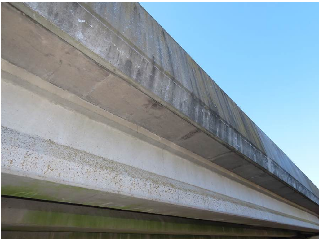
Photo 11: Underside of span 2 north deck overhang looking west. Transverse cracks with light efflo. Above, parapet with moisture staining and map cracking with light efflo.
