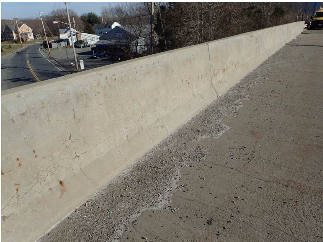
Photo 6: Span 2 North Parapet inside face looking east, typical condition of cracking and rust staining.
