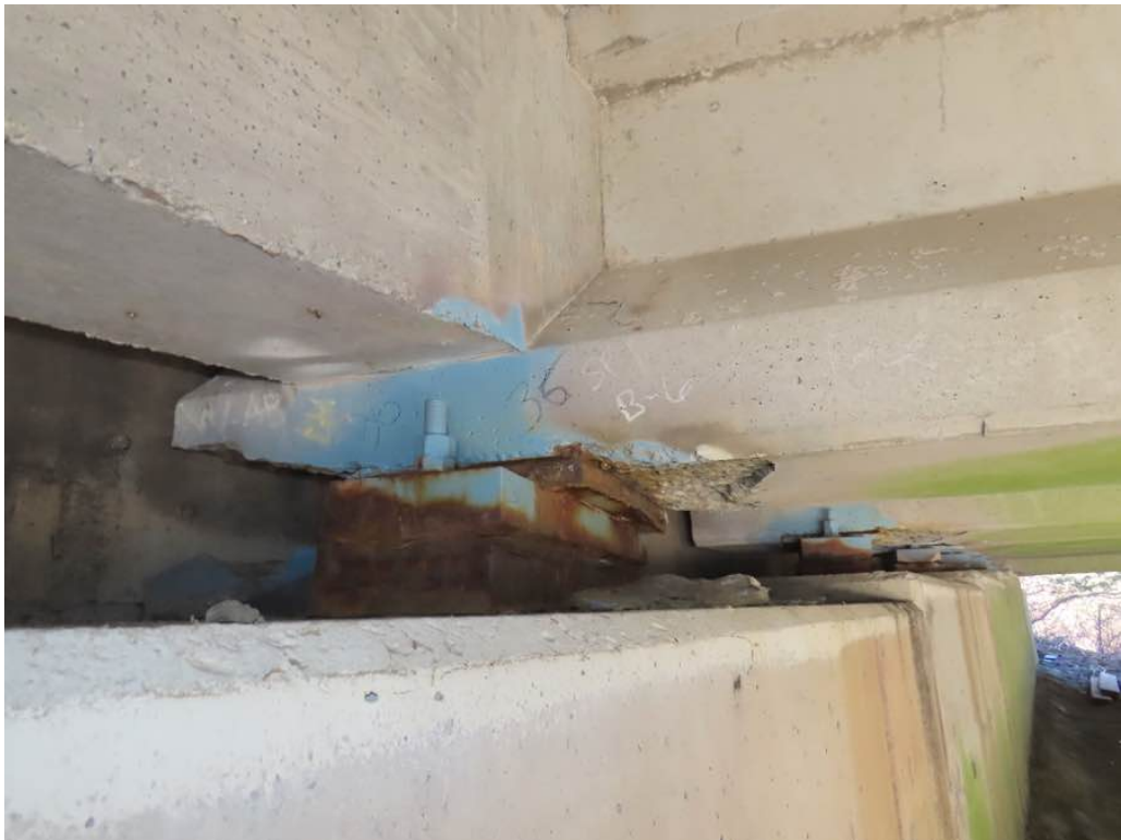
Photo 16: Beam 36, south face at the west abutment with spalls before and behind the bearing. Beam 35 in the background - Typical.
