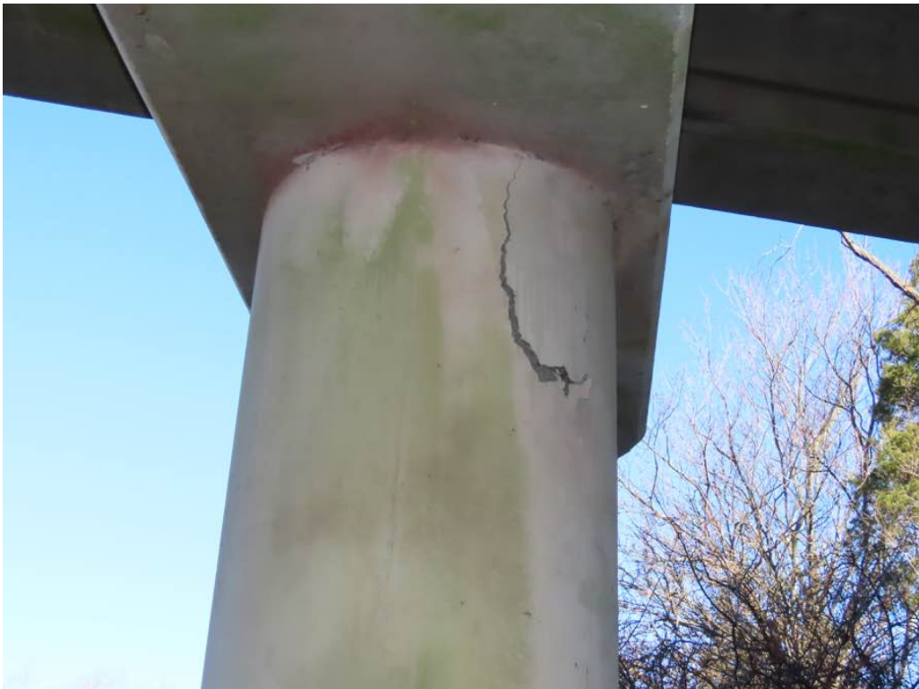
Photo 34: Pier 2, column 1, south face with a delam at the top.
