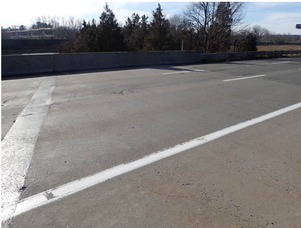
Photo 1: Span 1 looking south, typical condition with cracking, wheel rutting, and partially patched potholes.
