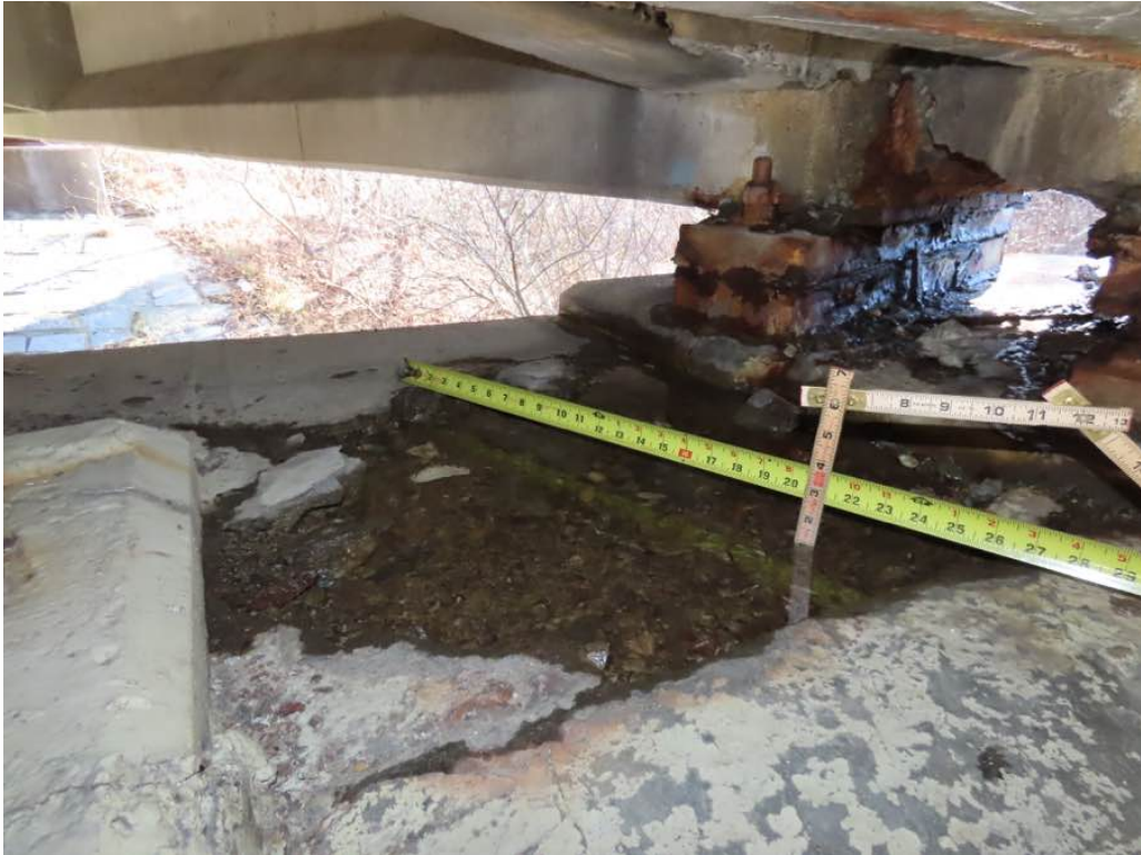
Photo 33: Top of pier 2 cap at bay 9 spall/scale is filled with water.
