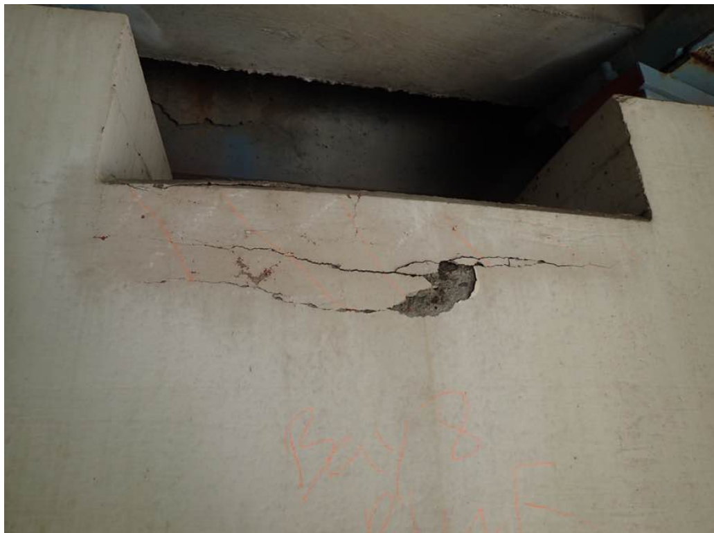
Photo 20: Pier 1 west face below Bay 8, spall/delamination.
