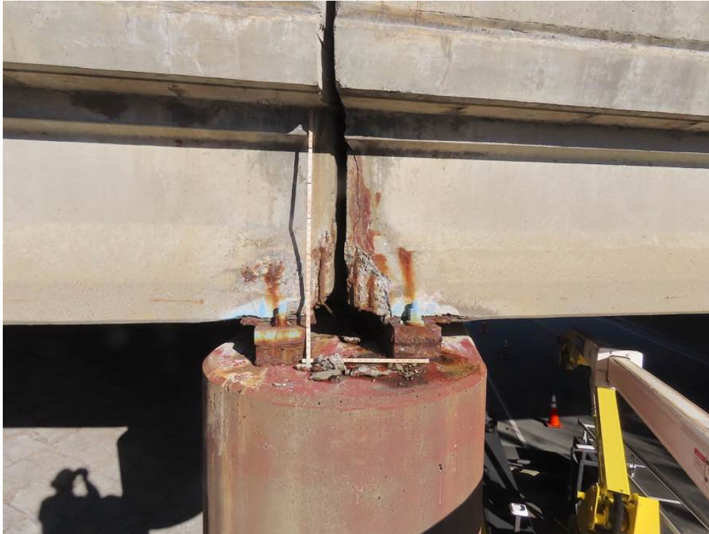
Photo 23: Beam ends 40 and 50 (L to R) south face at pier 1. Both with spalls with exposed corroded rebar and rust bleed. In addition, beam 50 with a vertical crack up to the top.
