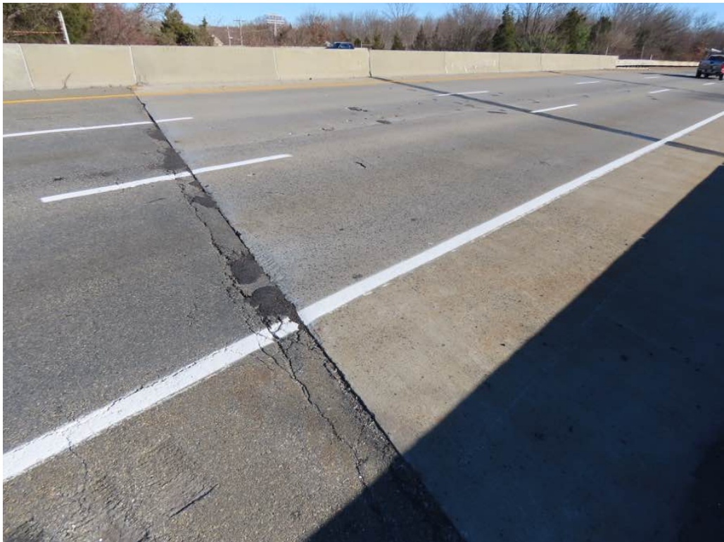
Photo 2: Overview of the full depth concrete deck and wearing surface looking east. Span 1 is in the foreground. On the left is the west approach pavement with curb to curb cracking and settlement.
