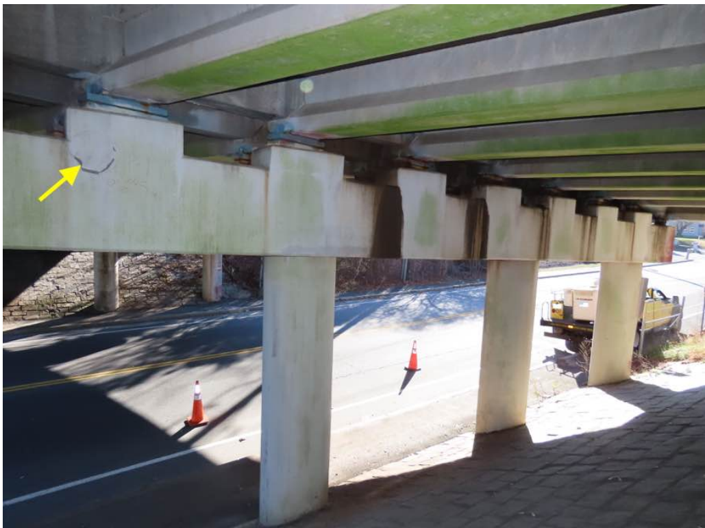
Photo 26: Overview of pier 1 west face with areas of water staining looking south. In the foreground, isolated delam (Y) below beam 33.
