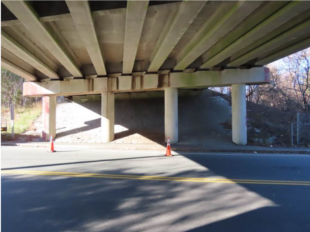
Photo 27: Overview of pier 1 east face with areas of water staining.
