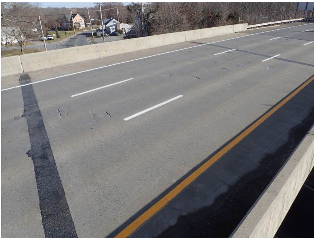
Photo 2: Spans 2 and 3 looking east, typical condition with cracking, wheel rutting, and partially patched potholes.
