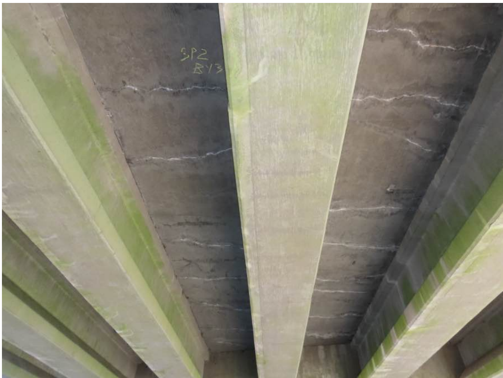
Photo 9: Close up of previous photo - Span 2 looking east, bays 3 and 4 (L to R) with transverse HL with light efflo - Typical.
