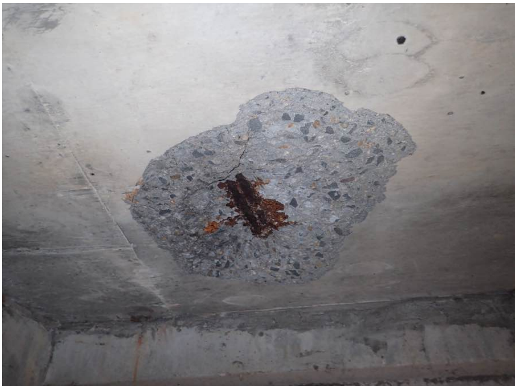
Photo 5: Span 3 Bay 5 at the East Abutment, spall with exposed rebar.
