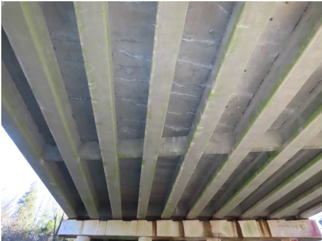
Photo 8: General underside of span 2 looking east, bays 1 through 9 (L to R). Bays with transverse cracks and efflo.
