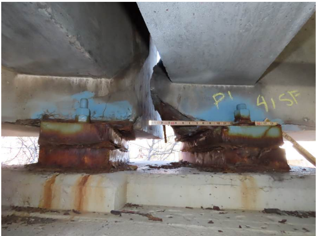
Photo 18: Close up of previous photo - Beam ends 31 and 41 south face at pier 1. Beam 31 with cracks and delams, beam 41 with end spall with exposed rebar - Typical.
