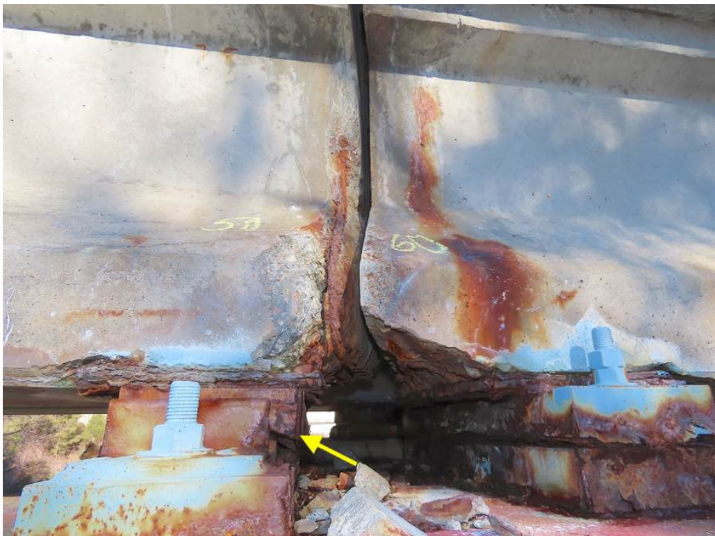
Photo 25: Beam ends 50 and 60 (L to R) south face at pier 2. Both with spalls with exposed corroded rebar and rust bleed. Beam 50 with expanded bearing (Y).
