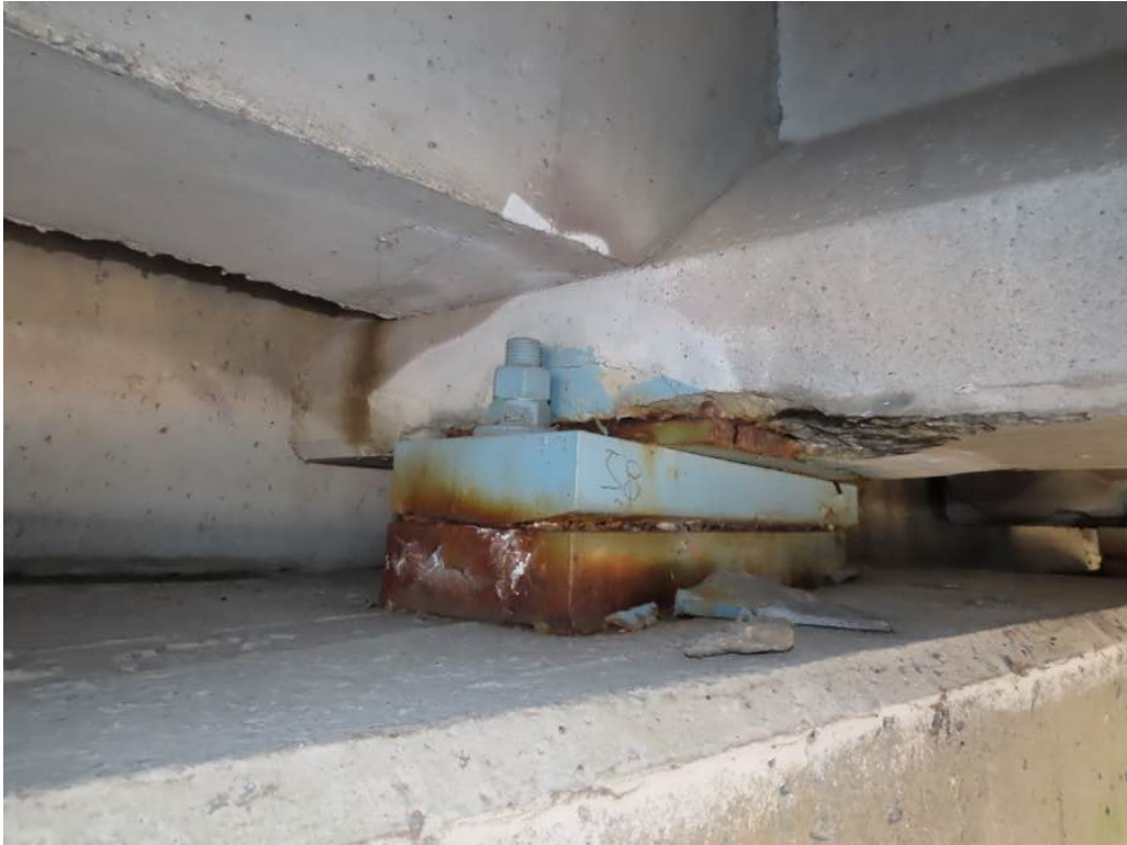
Photo 21: Beam 58, north face at the east abutment with spalls before the bearing - Typical.
