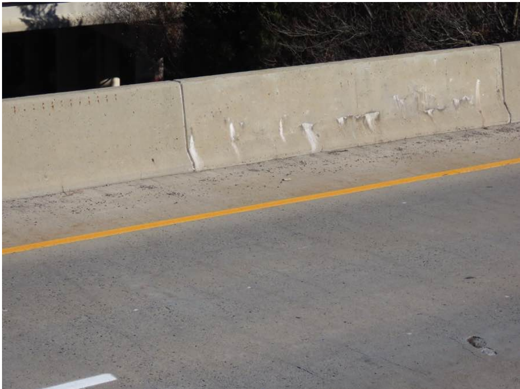
Photo 12: Span 2 parapet section near midspan with horizontal cracking with light to moderate efflo.
