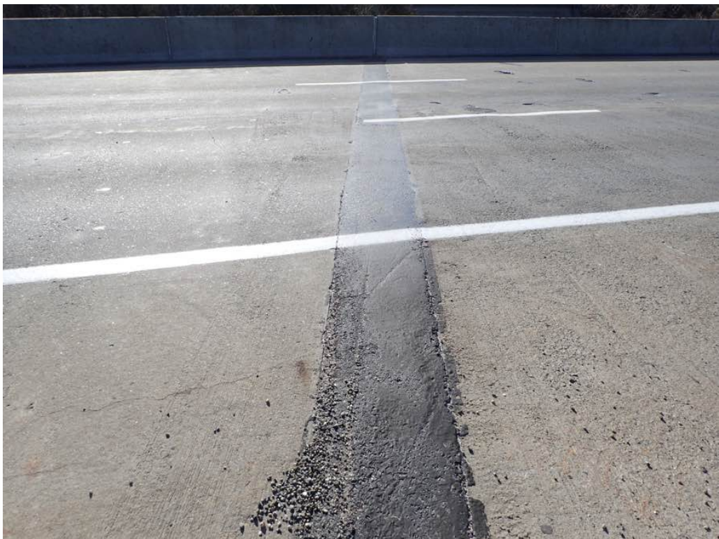
Photo 7: Pier 2 Deck Joint looking south, typical condition with adhesion separations.
