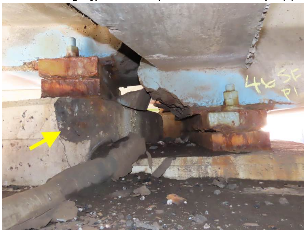
Photo 20: Beam ends 36 and 46 south face at pier 1. Beam 46 with end spall with exposed rebar and delam in front of bearing - Typical. Beam 36 pedestal with SE corner spall (Y).
