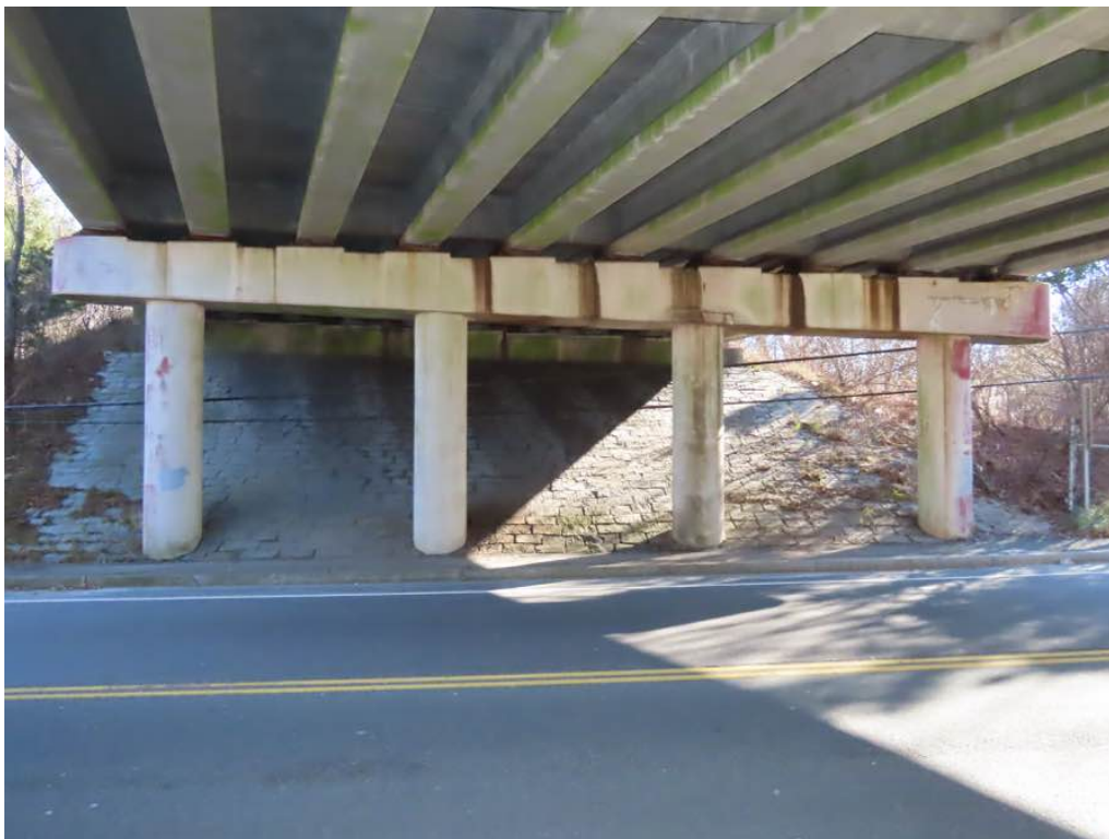
Photo 30: Overview of pier 2 west face with areas of water staining and HL cracking.
