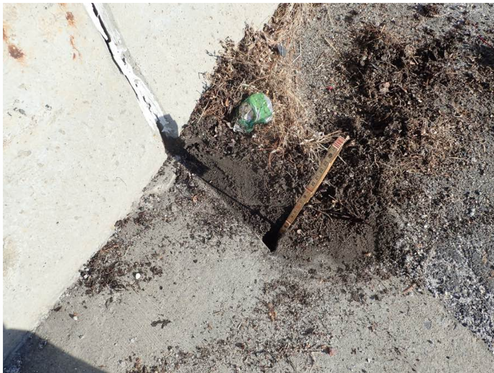
Photo 11: Northeast Corner, cutout with debris.
