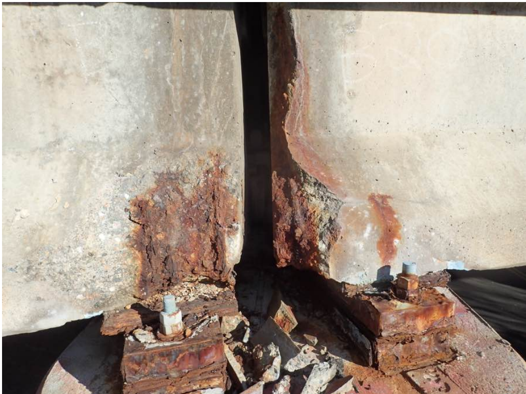
Photo 16: Beams 10 and 20 at Pier 1 south face, spalling with exposed rebar.
