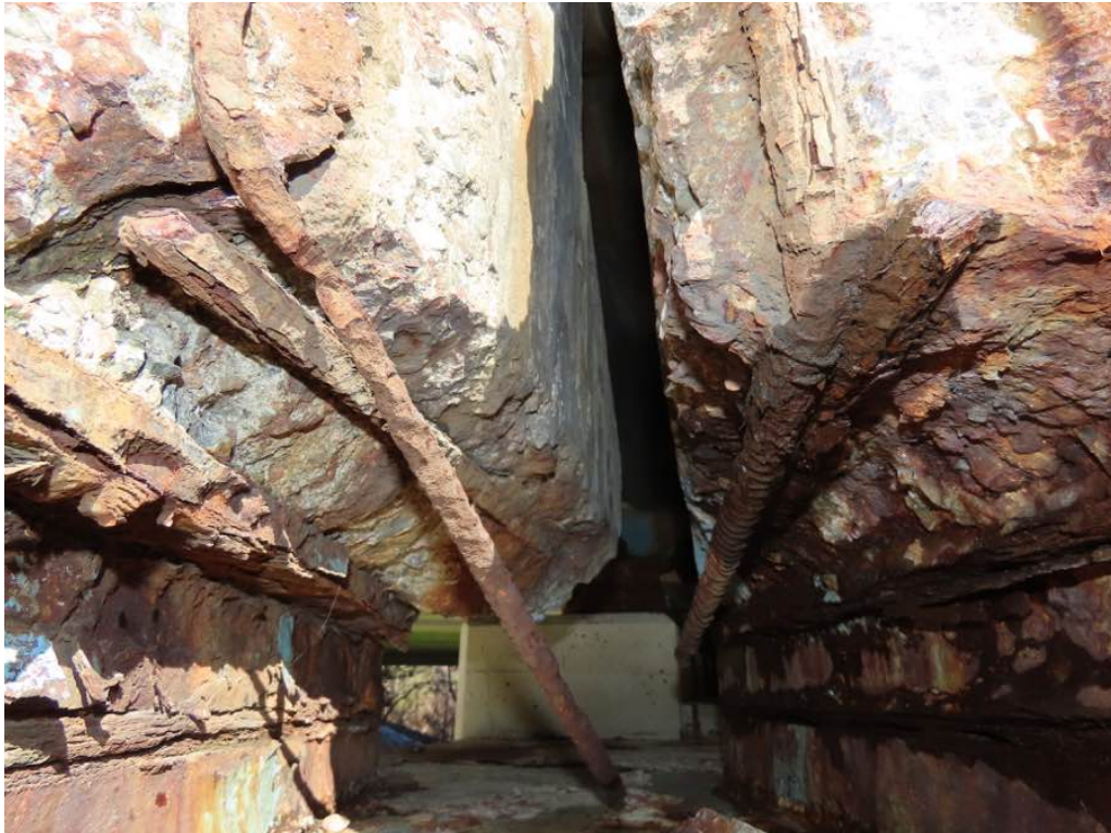
Photo 24: Close up of previous photo - Beam ends 40 and 50 (L to R) at pier 1 looking north. Both with end spalls with exposed corroded rebar.
