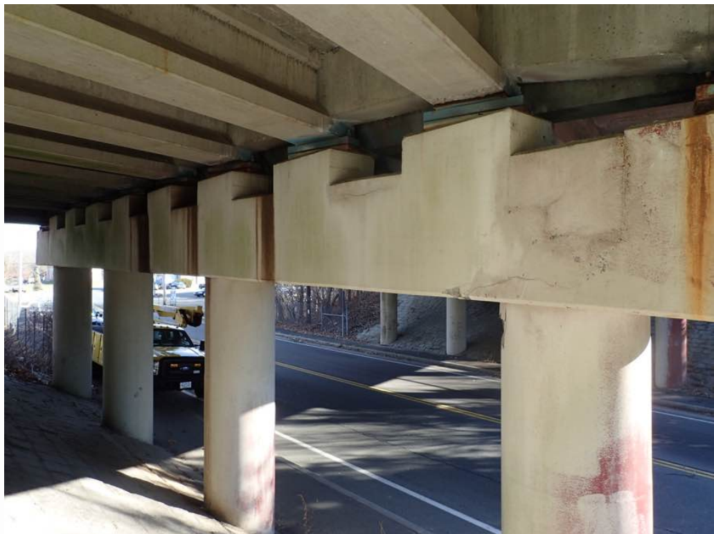
Photo 19: Pier 1 east face, typical condition with cracking and rust staining.
