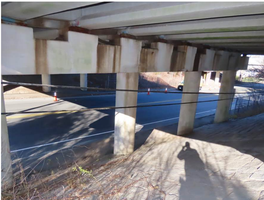
Photo 29: Overview of pier 2 east face with areas of water staining and HL cracking looking north.
