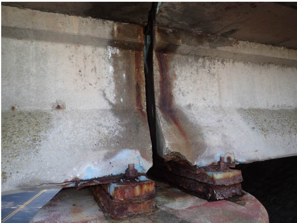
Photo 15: Beam 1 and 10 at Pier 1 north face, spalling and cracking past the bearing.
