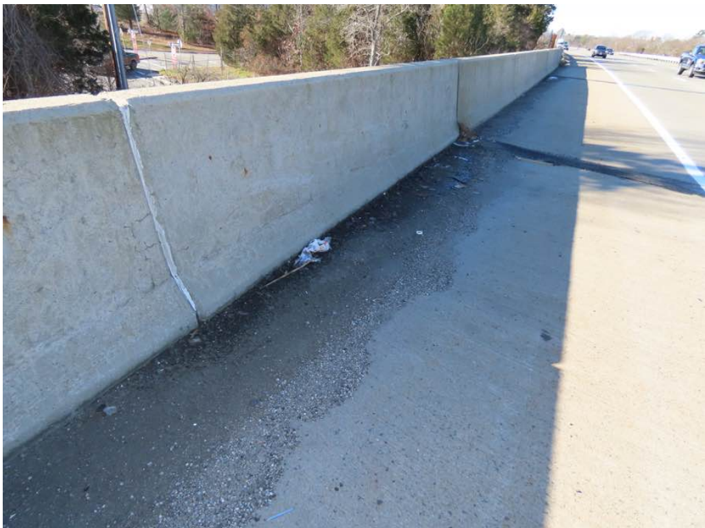
Photo 6: Overview ponding and debris along the south shoulder looking west.
