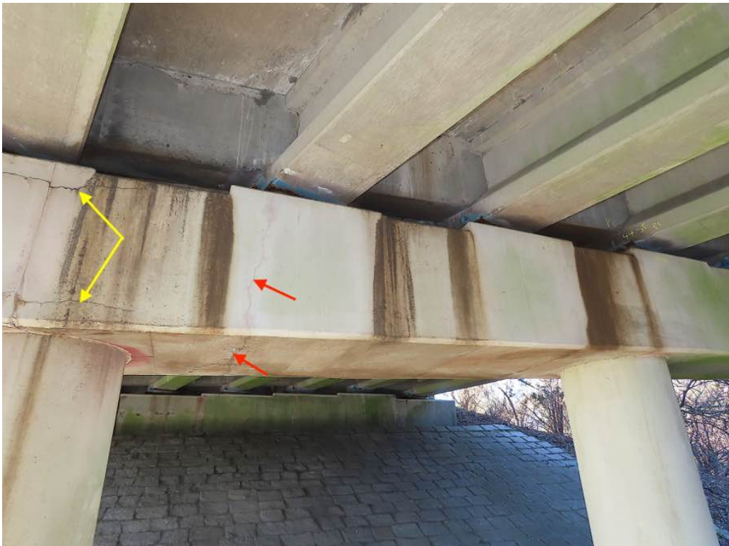
Photo 28: Close up of previous photo - Pier 1 cap with a vertical crack (R) on east face and transverse (R) along the underside of cap. To the left horizontal cracking (Y) at column 3.
