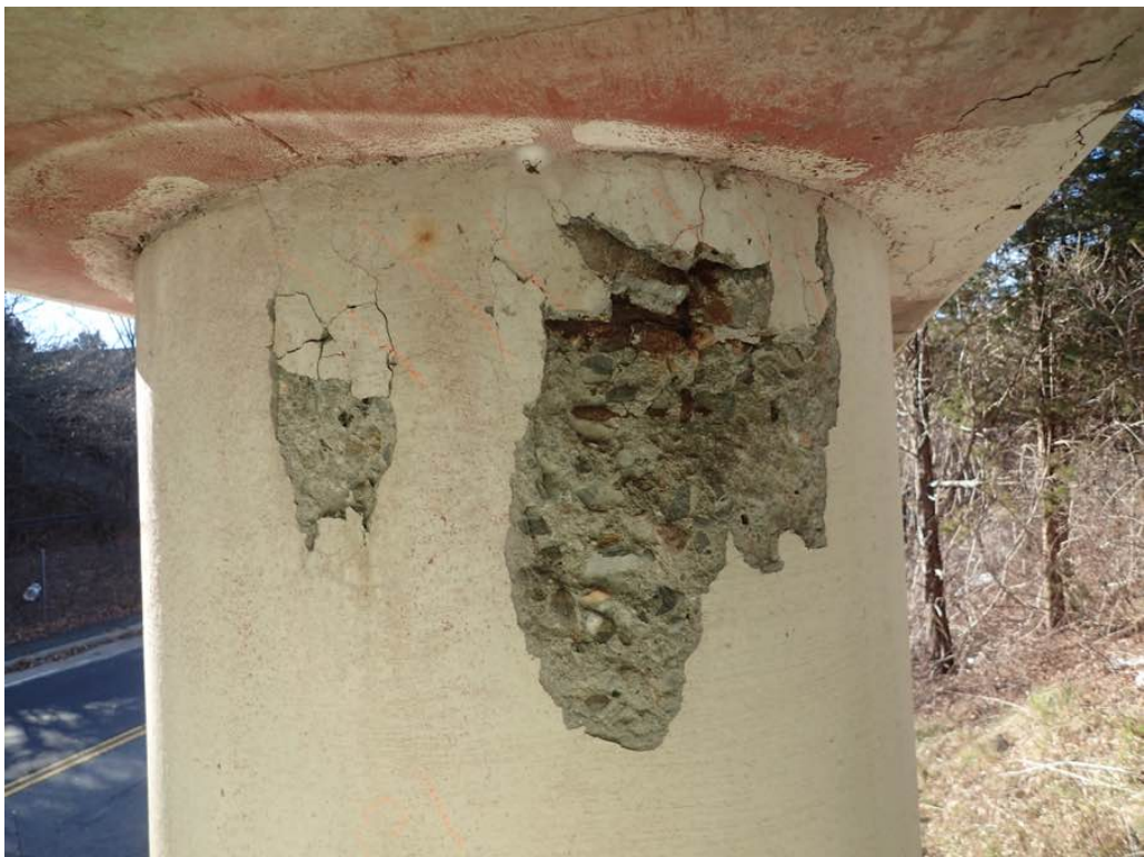
Photo 22: Pier 1 Column 4 north face, spall/delamination with exposed rebar.
