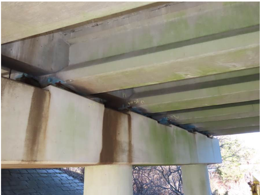
Photo 17: Overview of beam ends along the east face of pier 1 looking north.
