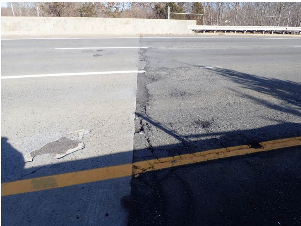
Photo 9: East Abutment looking north, approach pavement breaking up.
