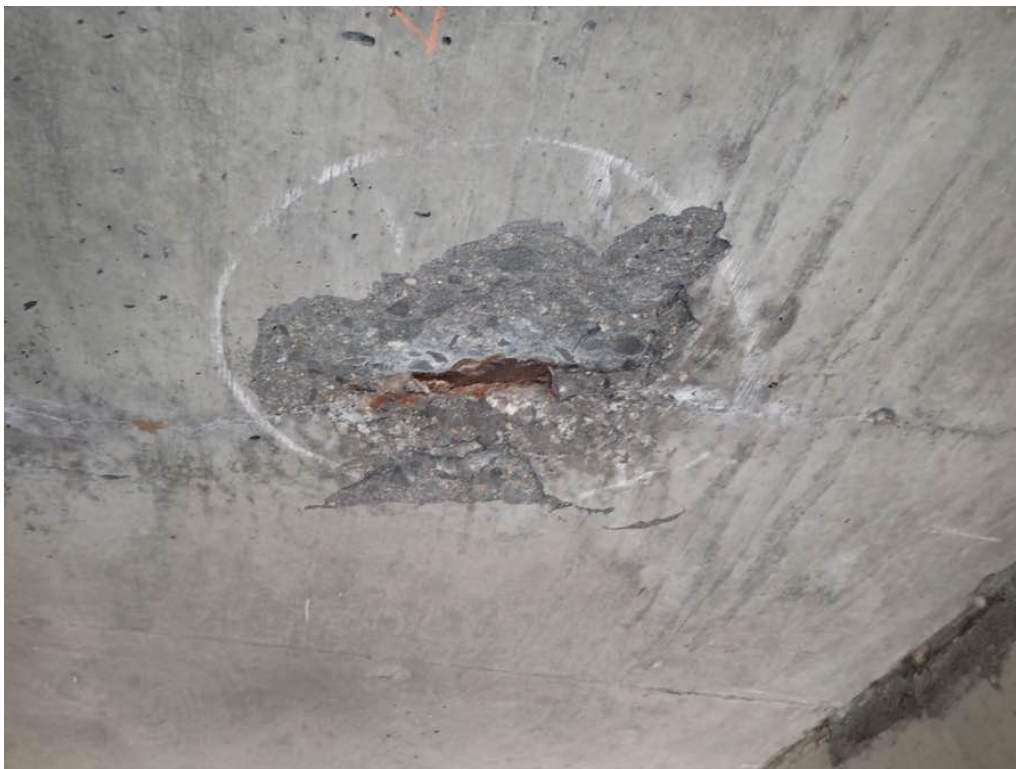
Photo 4: Span 2 Bay 9 over the southbound roadway, spall/delamination with exposed rebar.
