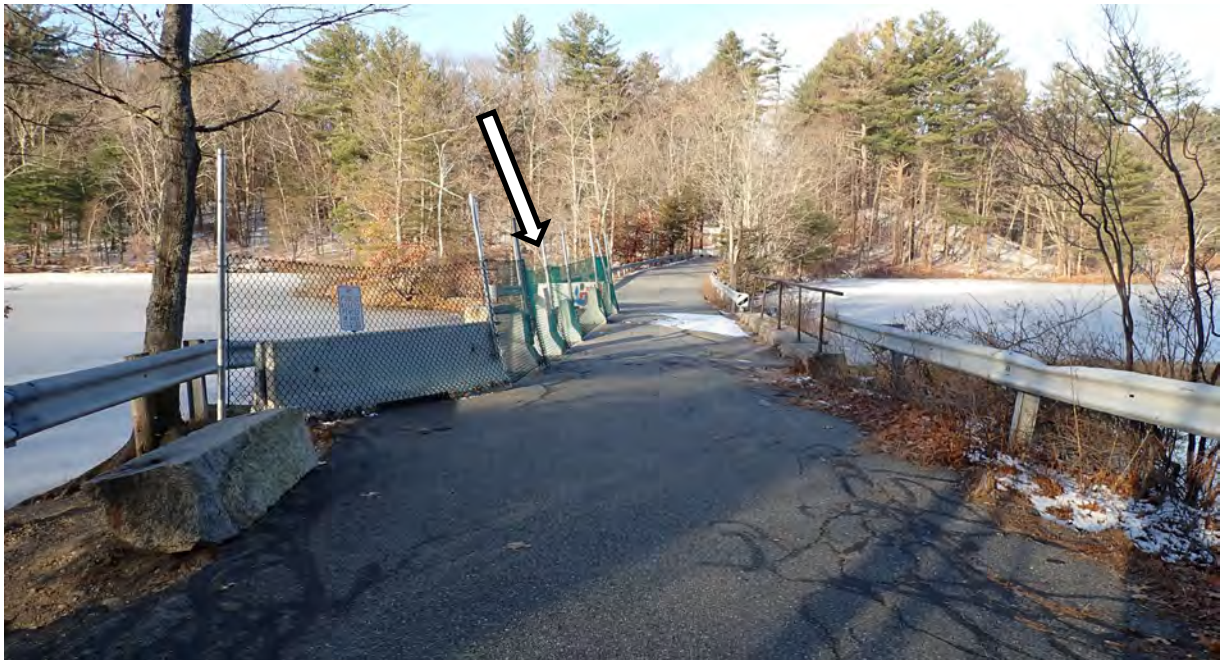
Photo #1: View northwest of Plummer Spring Rd, Newburyport facing Middle St, West Newbury over the Upper Artichoke Reservoir. Arrow indicates the failed section at the southern end of the roadway, directly over the bridge which is closed for public safety.
