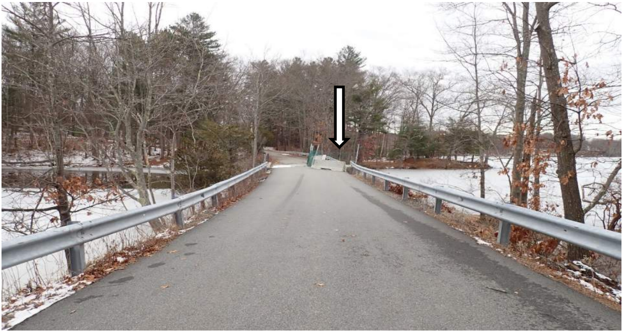
Photo #5: View southeast of Middle St, West Newbury facing Plummer Spring Rd, Newburyport over the Upper Artichoke Reservoir. Arrow indicates the failed section at the southern end of the roadway, directly over the bridge which is closed for public safety.
