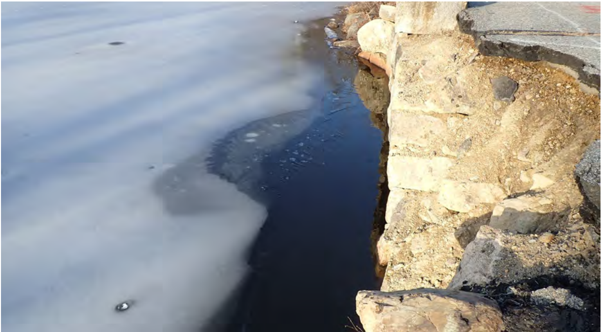
Photo #4: View northwest of Plummer Spring Rd, Newburyport facing Middle St, West Newbury over the Upper Artichoke Reservoir.. Up close view of the bridge in disrepair.
