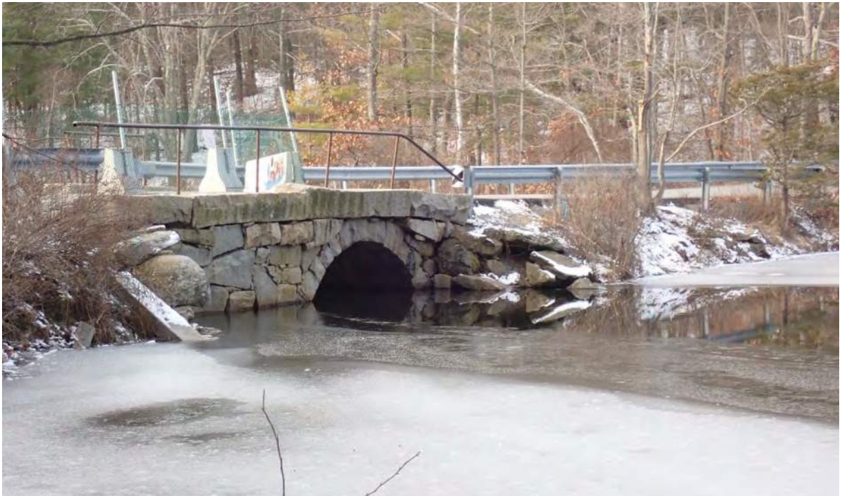
Photo #6: View southwest of the northern side of the roadway and bridge over the Upper Artichoke Reservoir.
