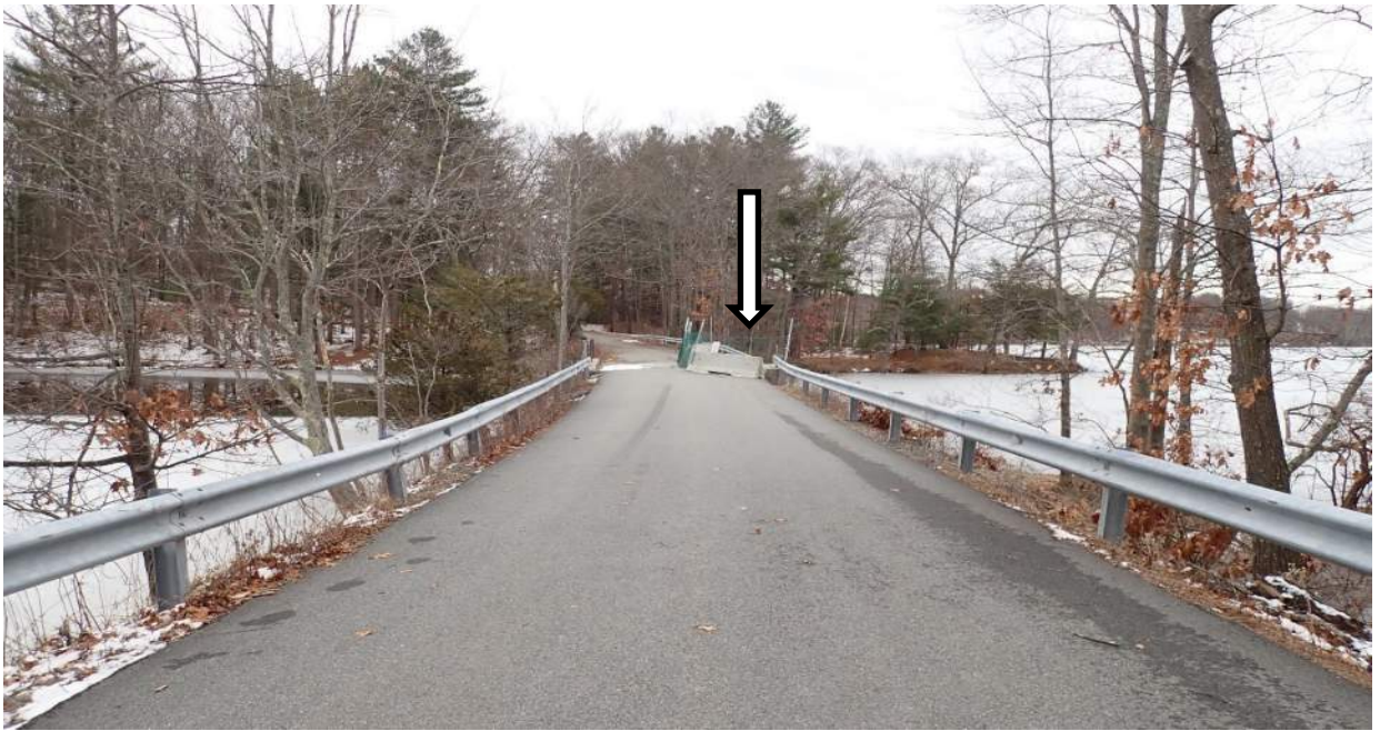
Photo #5: View southeast of Middle St, West Newbury facing Plummer Spring Rd, Newburyport over the Upper Artichoke Reservoir. Arrow indicates the failed section at the southern end of the roadway, directly over the bridge which is closed for public safety.
