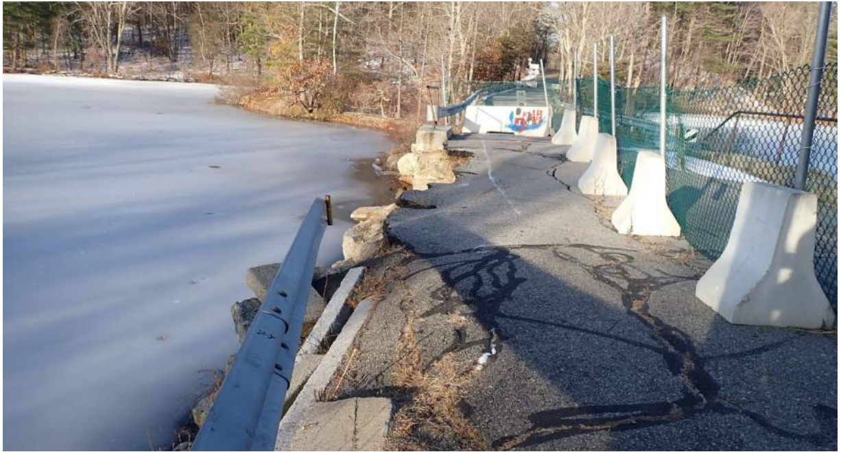
Photo #3: View northwest of Plummer Spring Rd, Newburyport facing Middle St, West Newbury over the Upper Artichoke Reservoir. View of the failed section at the southern end of the roadway, directly over the bridge which is closed for public safety.
