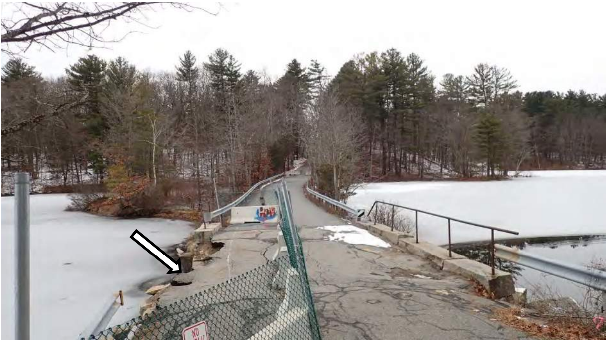
Photo #2: View northwest of Plummer Spring Rd, Newburyport facing Middle St, West Newbury over the Upper Artichoke Reservoir. Arrow indicates the failed section at the southern end of the roadway, directly over the bridge which is closed for public safety.
