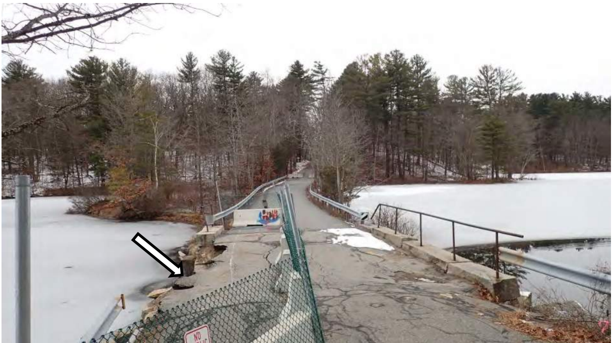
Photo #2: View northwest of Plummer Spring Rd, Newburyport facing Middle St, West Newbury over the Upper Artichoke Reservoir. Arrow indicates the failed section at the southern end of the roadway, directly over the bridge which is closed for public safety.
