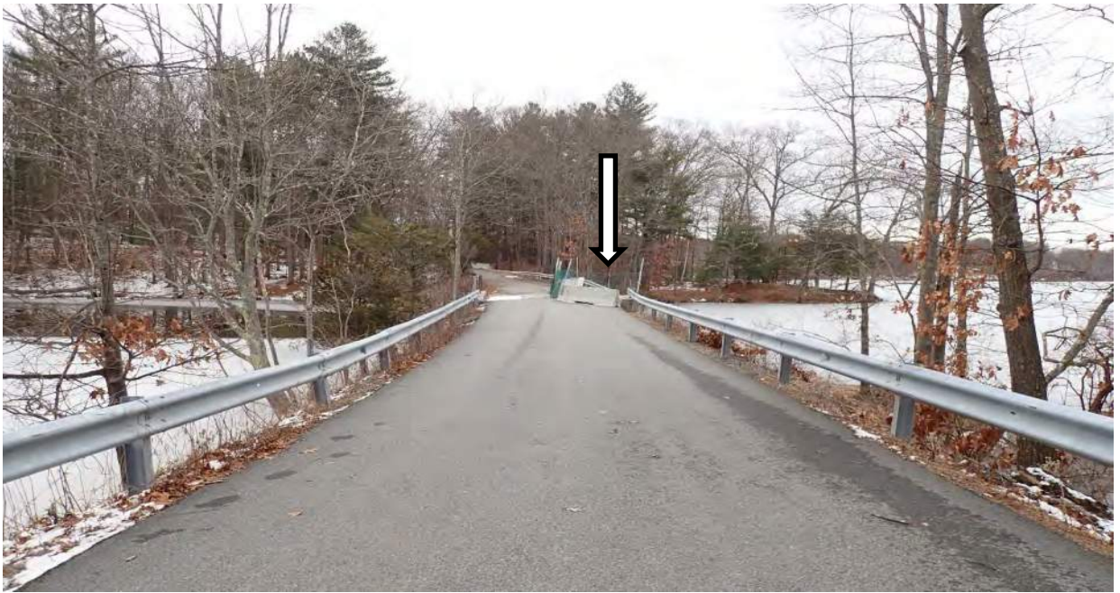
Photo #5: View southeast of Middle St, West Newbury facing Plummer Spring Rd, Newburyport over the Upper Artichoke Reservoir. Arrow indicates the failed section at the southern end of the roadway, directly over the bridge which is closed for public safety.
