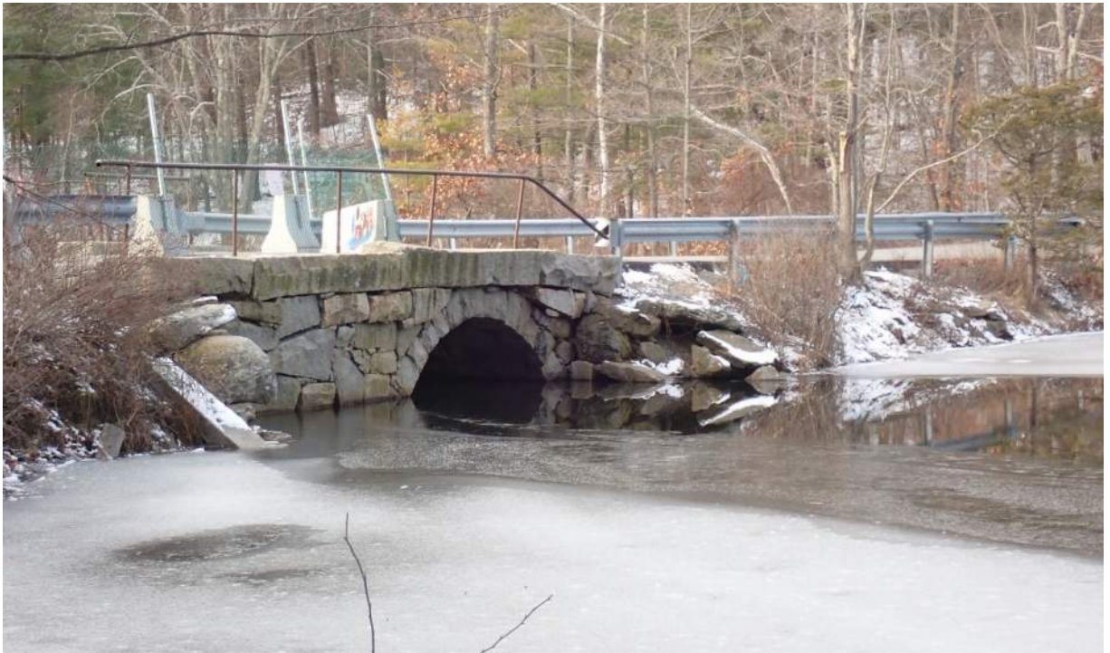
Photo #6: View southwest of the northern side of the roadway and bridge over the Upper Artichoke Reservoir.
