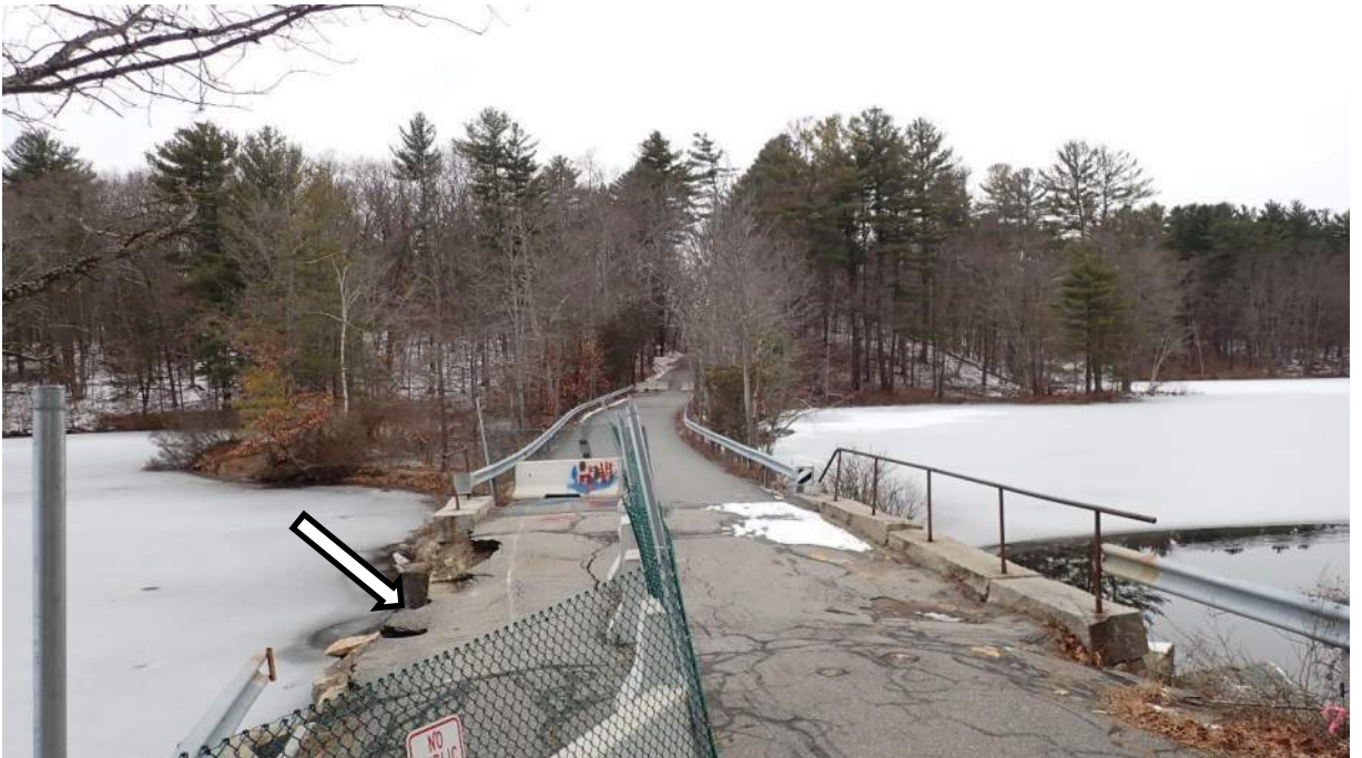
Photo #2: View northwest of Plummer Spring Rd, Newburyport facing Middle St, West Newbury over the Upper Artichoke Reservoir. Arrow indicates the failed section at the southern end of the roadway, directly over the bridge which is closed for public safety.
