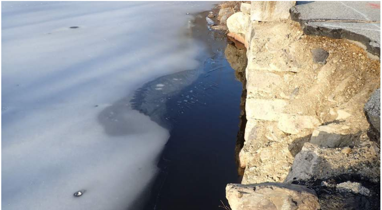
Photo #4: View northwest of Plummer Spring Rd, Newburyport facing Middle St, West Newbury over the Upper Artichoke Reservoir.. Up close view of the bridge in disrepair.
