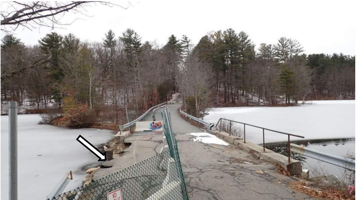
Photo #2: View northwest of Plummer Spring Rd, Newburyport facing Middle St, West Newbury over the Upper Artichoke Reservoir. Arrow indicates the failed section at the southern end of the roadway, directly over the bridge which is closed for public safety.
