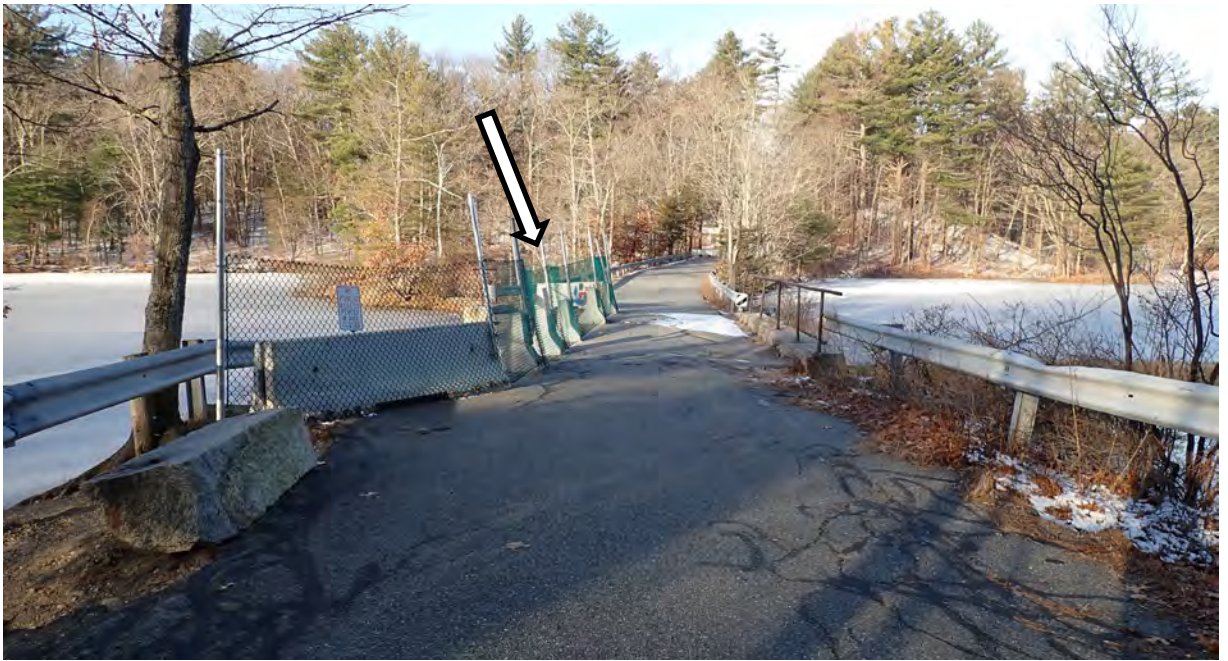
Photo #1: View northwest of Plummer Spring Rd, Newburyport facing Middle St, West Newbury over the Upper Artichoke Reservoir. Arrow indicates the failed section at the southern end of the roadway, directly over the bridge which is closed for public safety.
