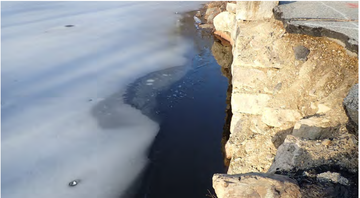
Photo #4: View northwest of Plummer Spring Rd, Newburyport facing Middle St, West Newbury over the Upper Artichoke Reservoir.. Up close view of the bridge in disrepair.
