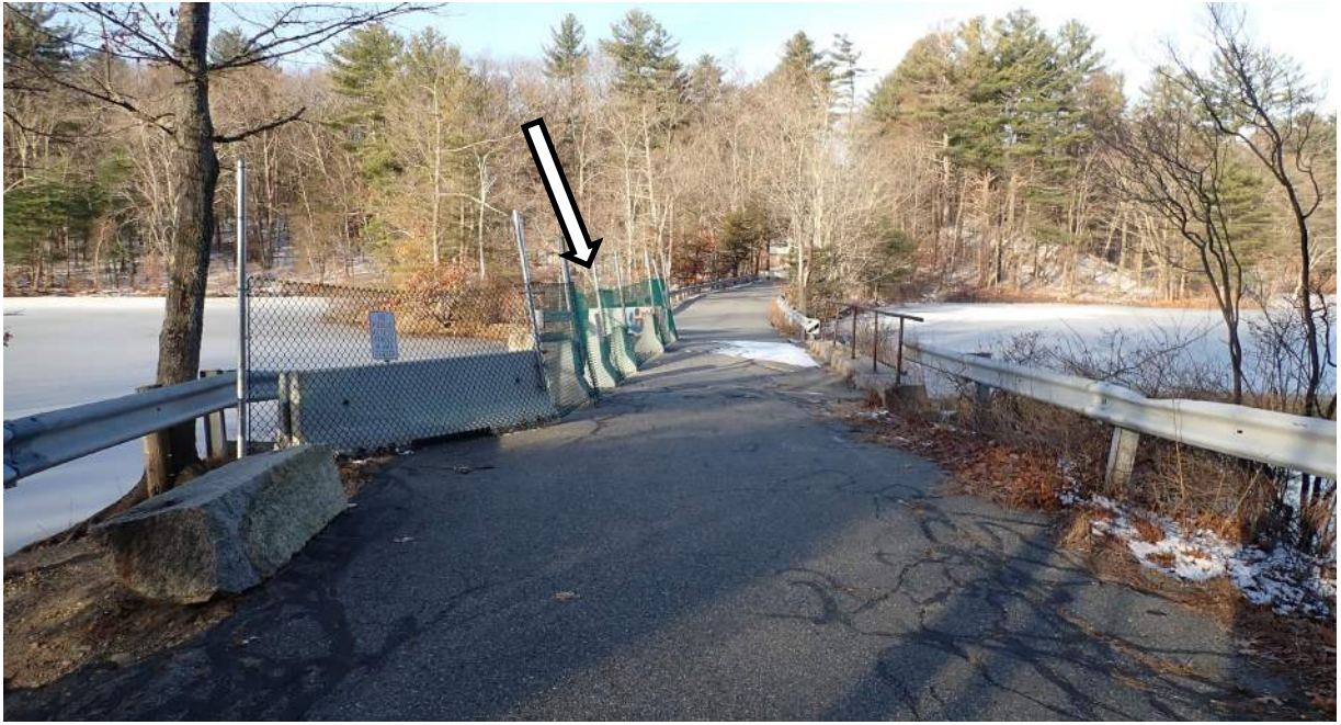
Photo #1: View northwest of Plummer Spring Rd, Newburyport facing Middle St, West Newbury over the Upper Artichoke Reservoir. Arrow indicates the failed section at the southern end of the roadway, directly over the bridge which is closed for public safety.
