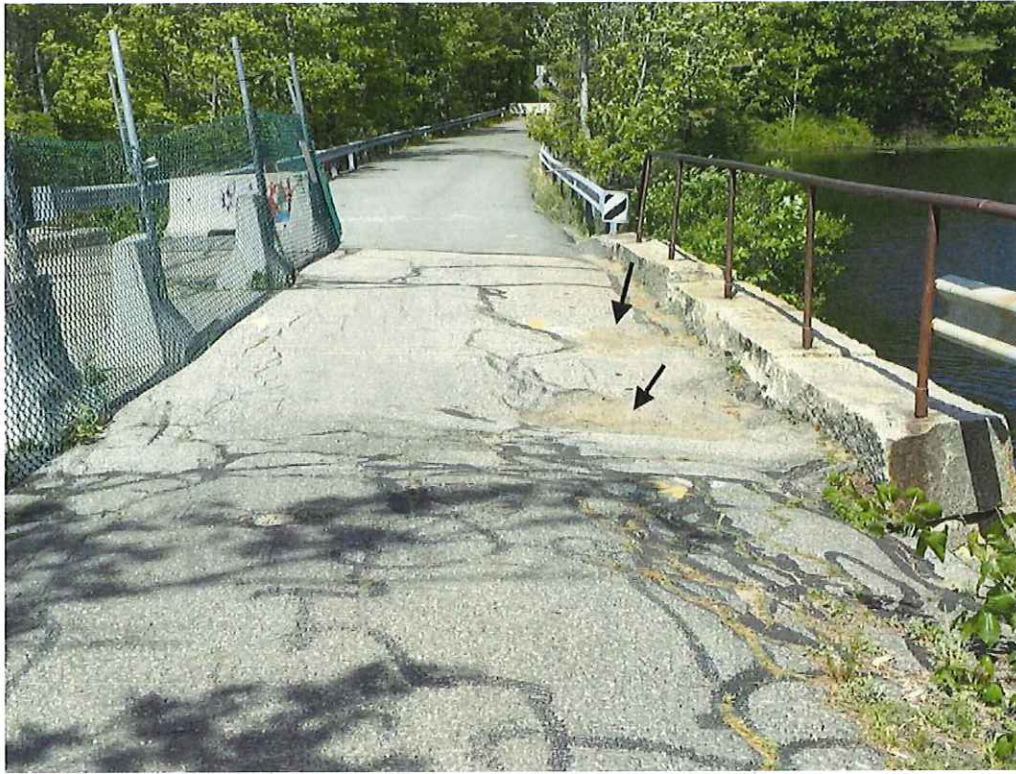
Photo 11: Areas of heavy settlement and depression along the north spandrel wall (heaviest at the East end) up to 1' deep. (Looking West).
