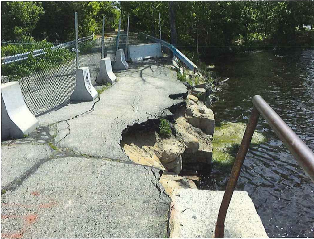
Photo 15: The collapsed area along the south side of the bridge. (Looking East).
