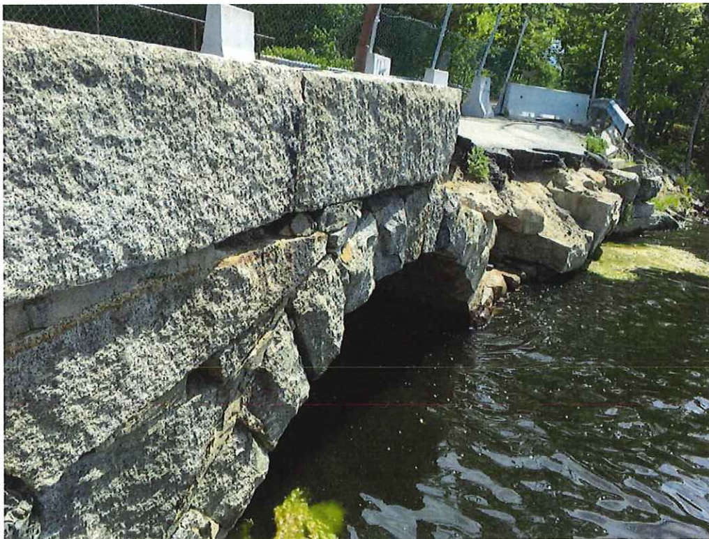
Photo 16: The collapsed spandrel wall along the south side of the bridge.
