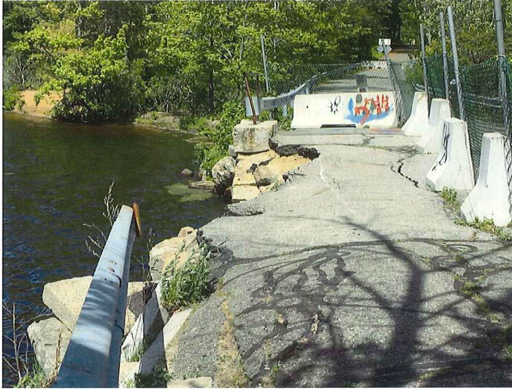
Photo 13: The collapsed area along the south side of the bridge. (Looking West).
