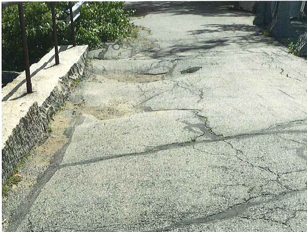
Photo 10: Areas of heavy settlement and depression along the north spandrel wall (heaviest at the East end) up to 1' deep. (Looking East).
