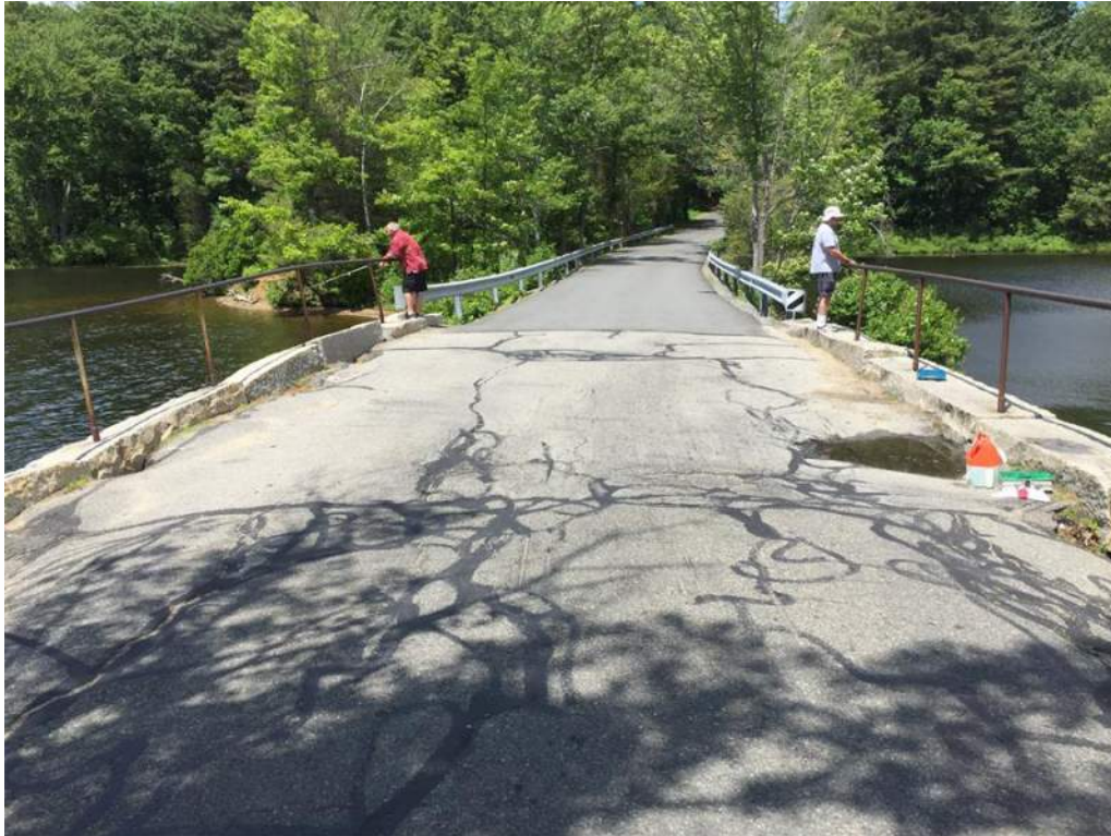
Photo 1: Bridge Bituminous Wearing Surface Crack Sealant Failure
