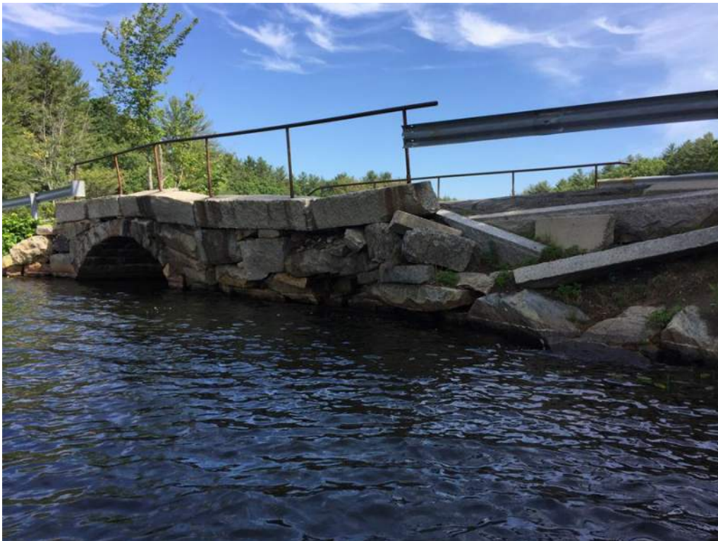
Photo 14: Southeast Bridge Rail/Curb Leaning Outwardly
