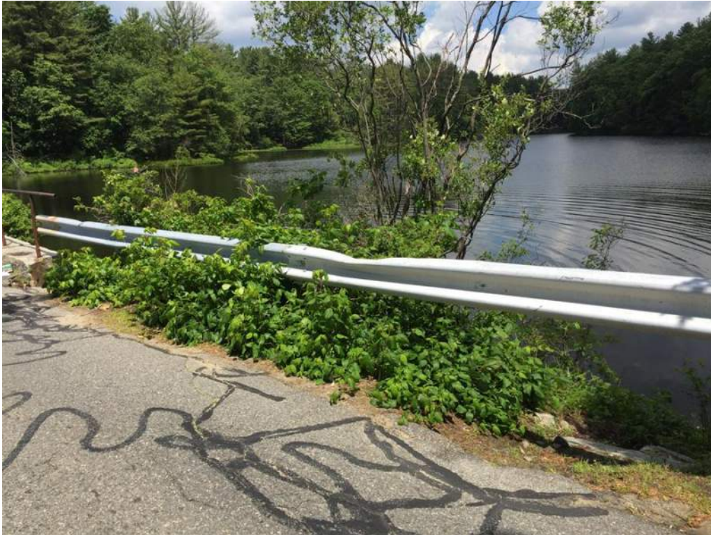
Photo 17: Southwest Approach Guardrail Minor Impact Damage
