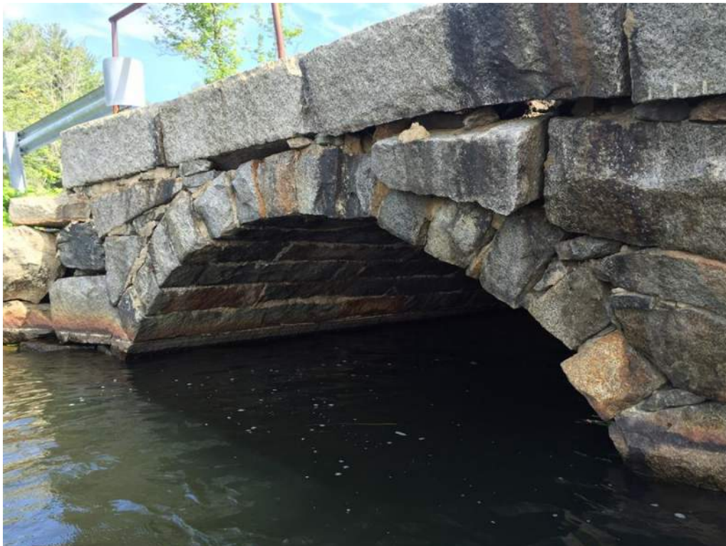
Photo 10: South Fascia Stone above Keystone Displacement
