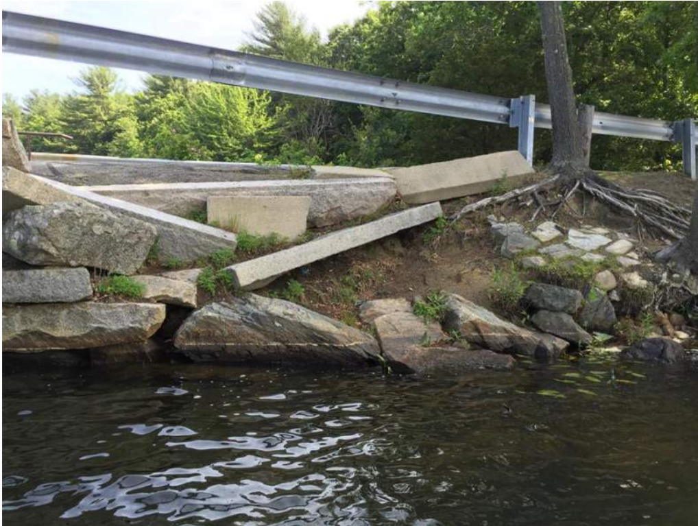
Photo 13: Southeast Wingwall End Displaced Curb Stones with Erosion
