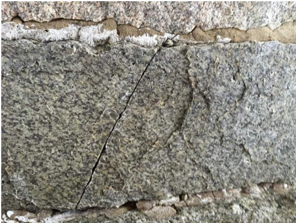
Photo 8: Arch Ring at Crown Approximately 10'-11" from South Fascia Crack in Stone
