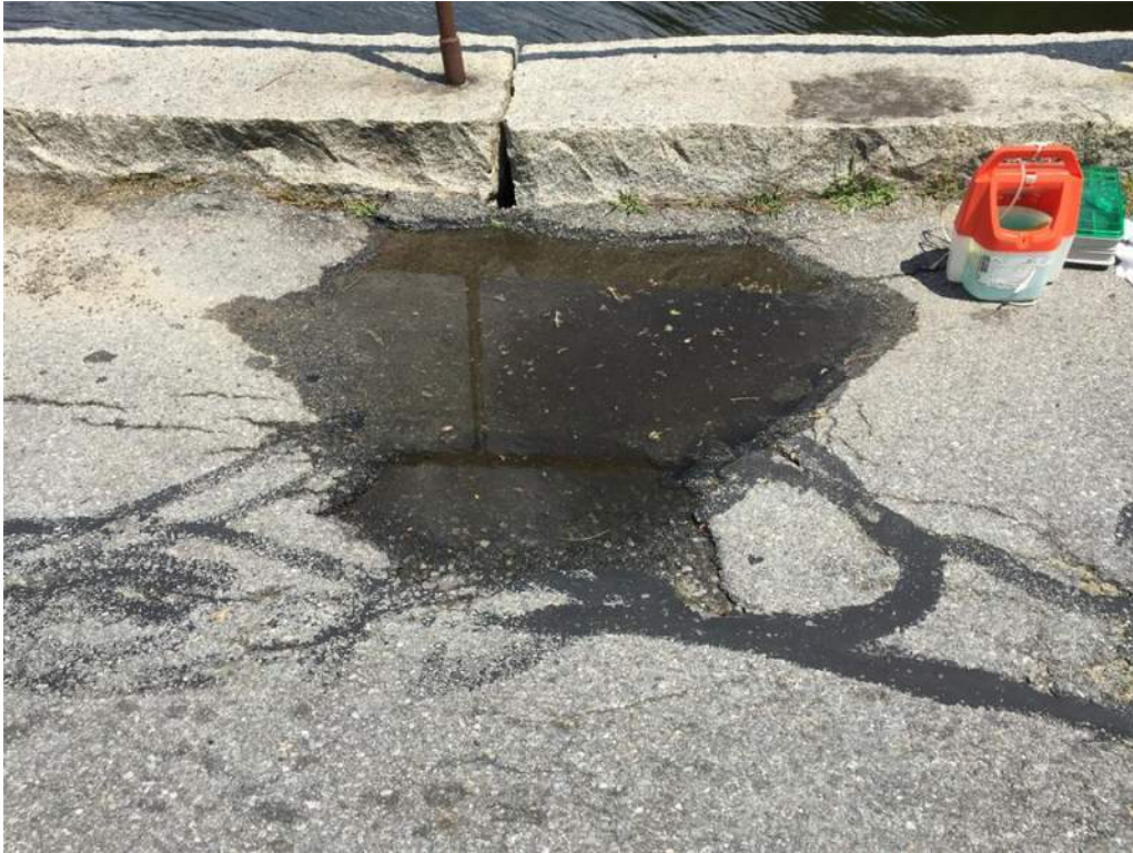
Photo 5: Northeast Approach Pavement Pothole
