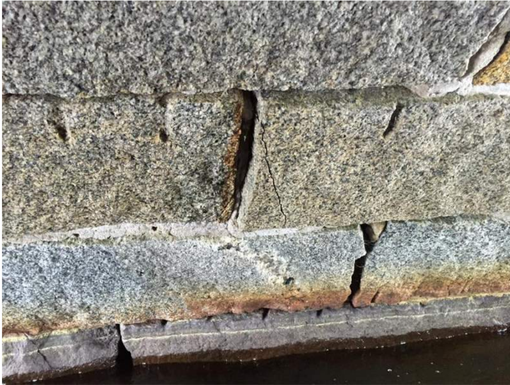
Photo 9: Arch Ring above East Spring Line Approximately 10'-11" from South Fascia Crack in Stone
