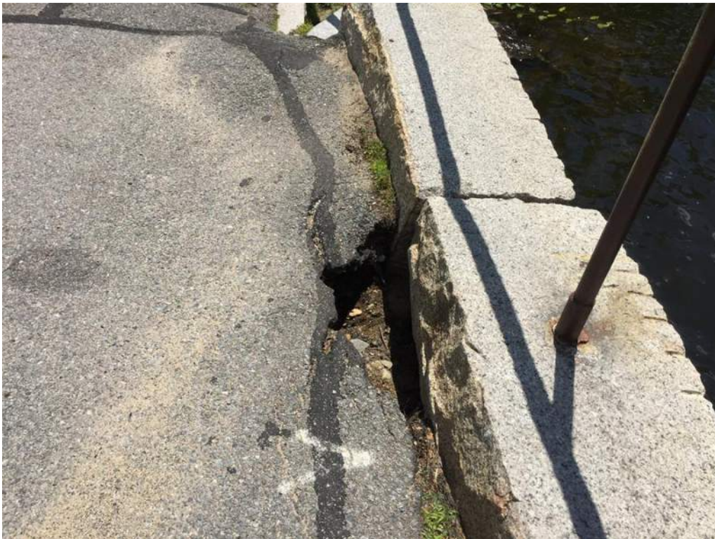
Photo 4: Southeast Approach Pavement Failed Pavement Voided Area
