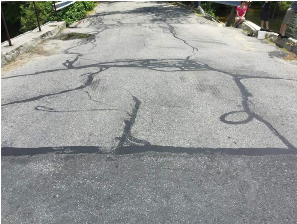
Photo 6: Southeast Approach Pavement Settlement
