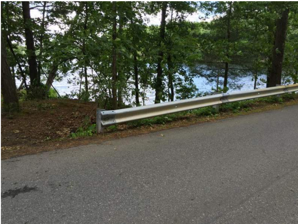
Photo 18: Southeast Approach Guardrail Terminates with Blunted End
