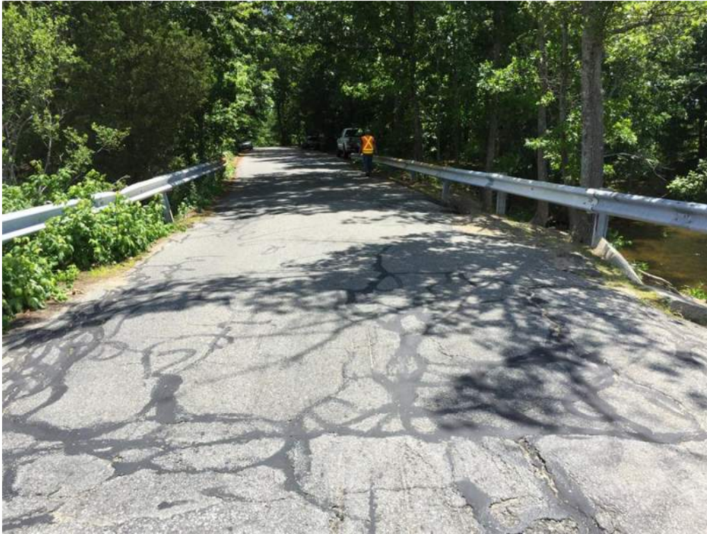
Photo 3: East Approach Pavement Map Cracking and Settlement
