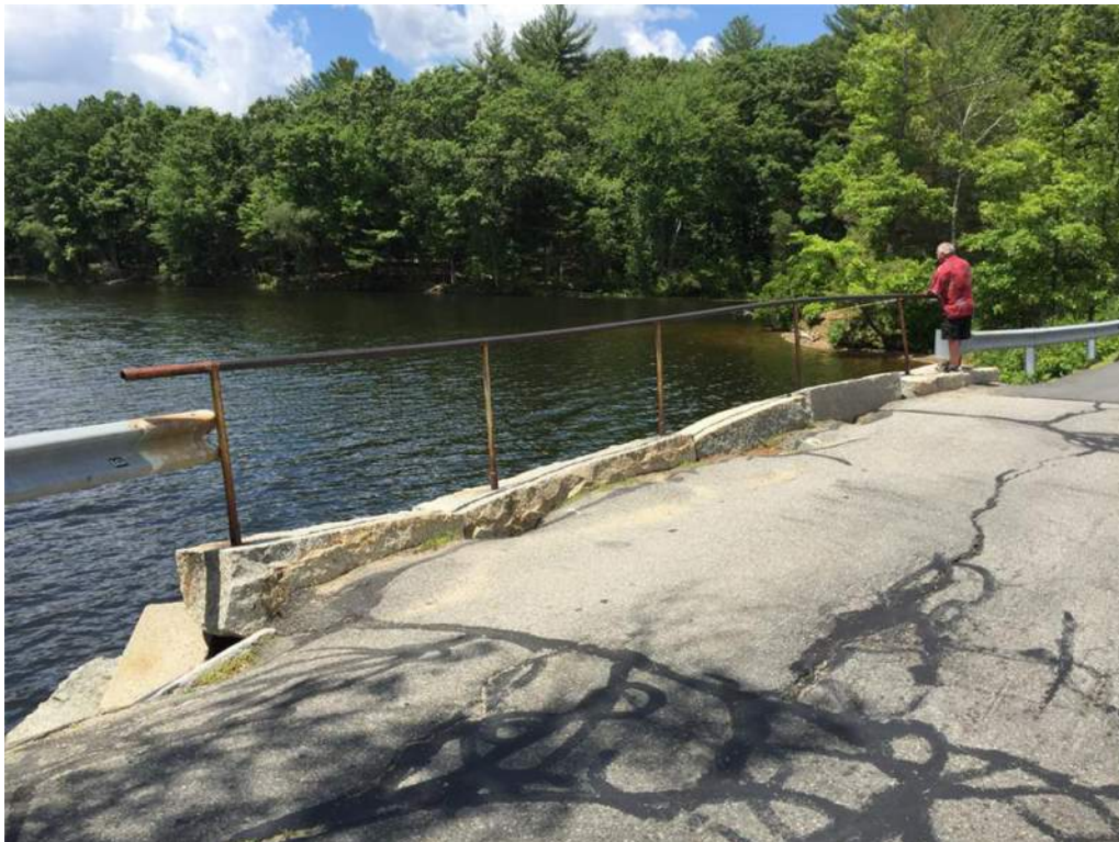
Photo 2: South Bridge Curb Displaced Outwardly up to 8"
