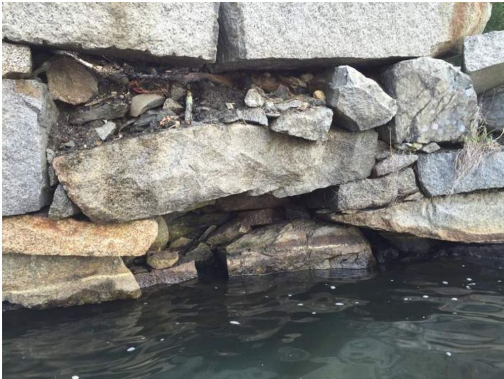
Photo 12: Southeast Wingwall Voided Areas of Missing Stones
