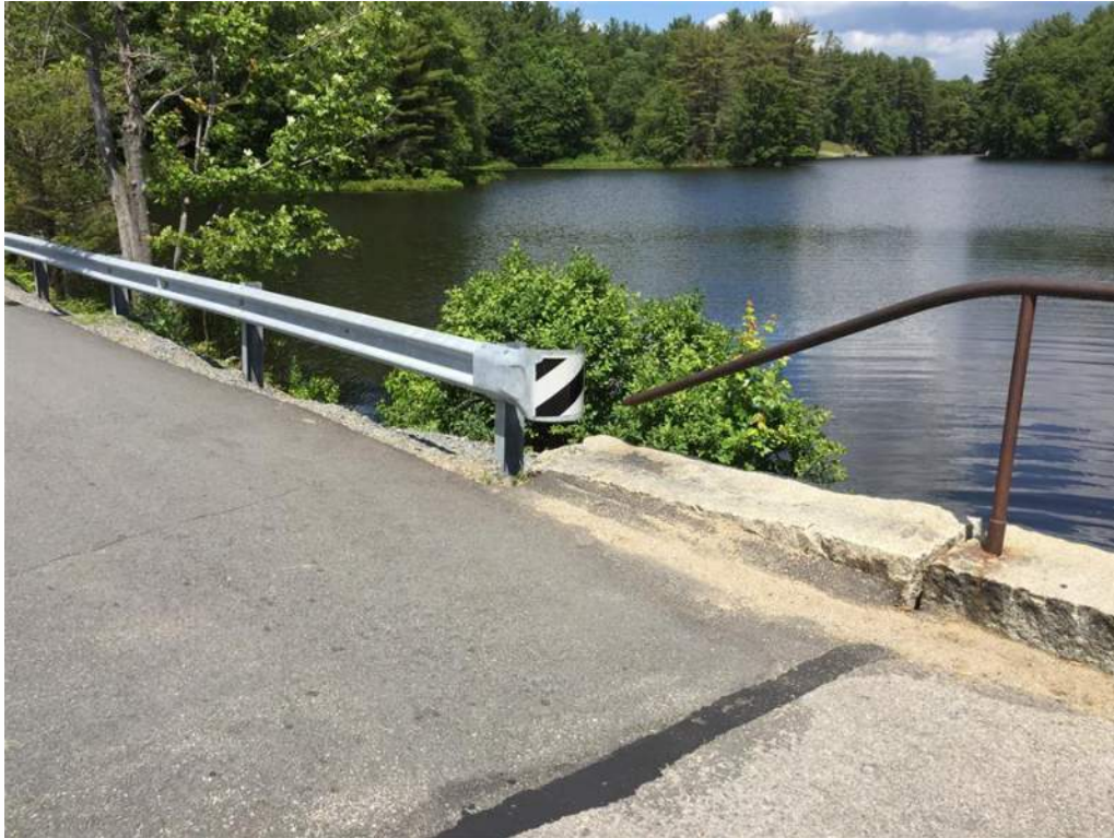
Photo 15: Northwest Bridge Rail End is Bent and Transition Rail Ends with Fisted End
