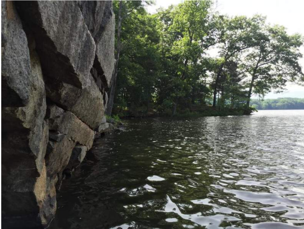
Photo 11: Southeast Wingwall Displacement up to 24"
