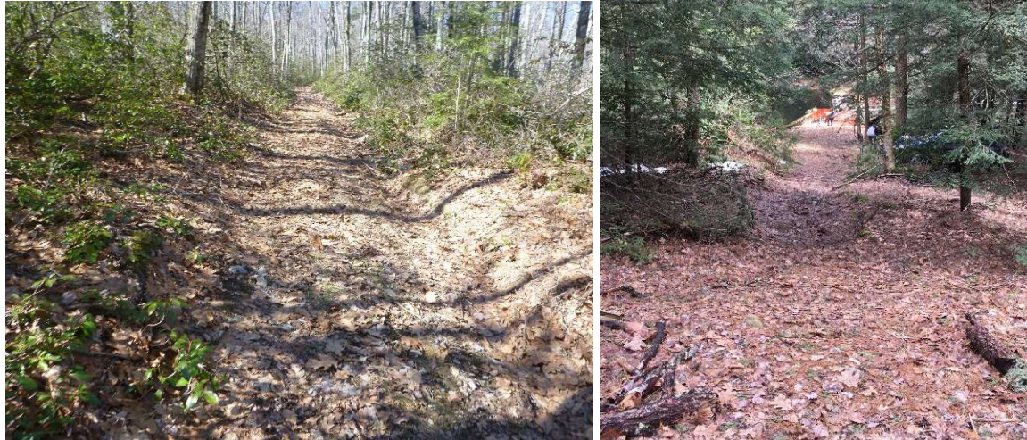
Figure 10. Existing dirt access road to be used during the removal of Becker Pond Dam (left) looking north along the road and (right) looking east towards the dam.
