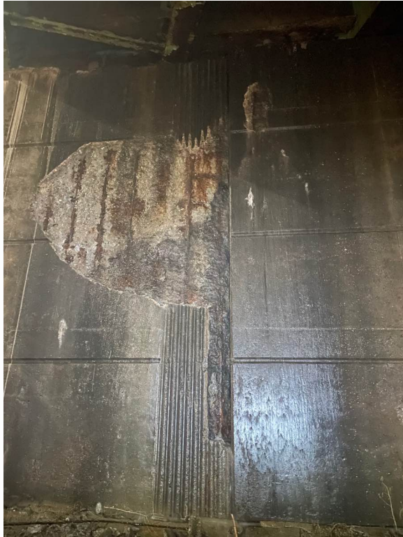
Photo 33: North abutment spall below Beam 202.
