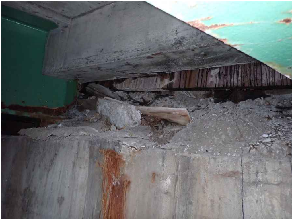
Photo 28: Typical debris on the South Abutment bridge seat.
