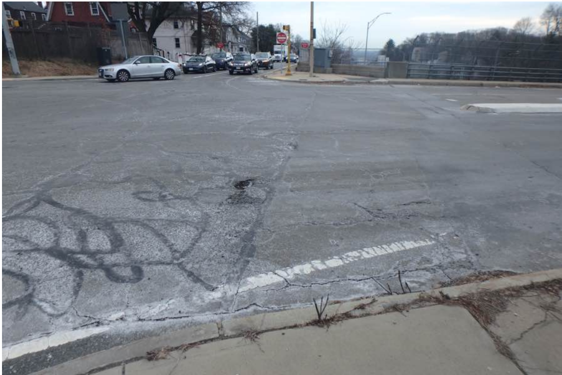
Photo 23: North approach roadway - typical severe map cracking throughout with potholes.
