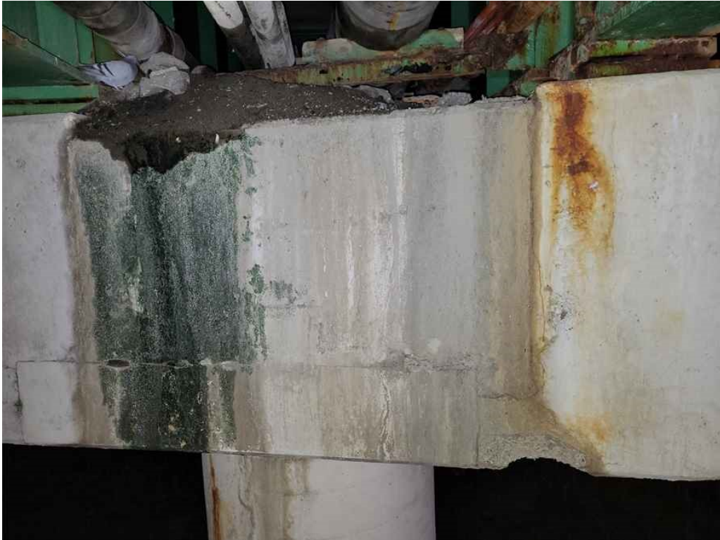
Photo 65: Pier cap, north face, bay 1, several full height vertical cracks x 1/16" wide throughout, rust staining under beam 8 and a corner spall at the bottom, 1' wide x 5" high x 4" deep.
