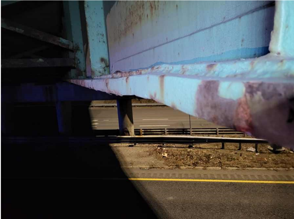
Photo 31: Girder 5, span 1: minor impact damage to the bottom flange at mid-span with minor bent of girder stiffener. Looking South).
