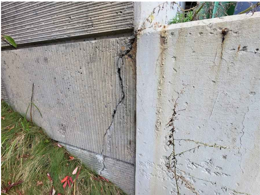
Photo 54: Northwest wingwall: full height vertical crack with minor spalling at the top corner, up to 1" wide.
