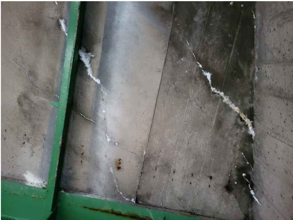
Photo 6: Deck ,Span 1, Bay 1: Multiple transverse hairline cracks with light efflorescence near south abutment, up to full bay width.
