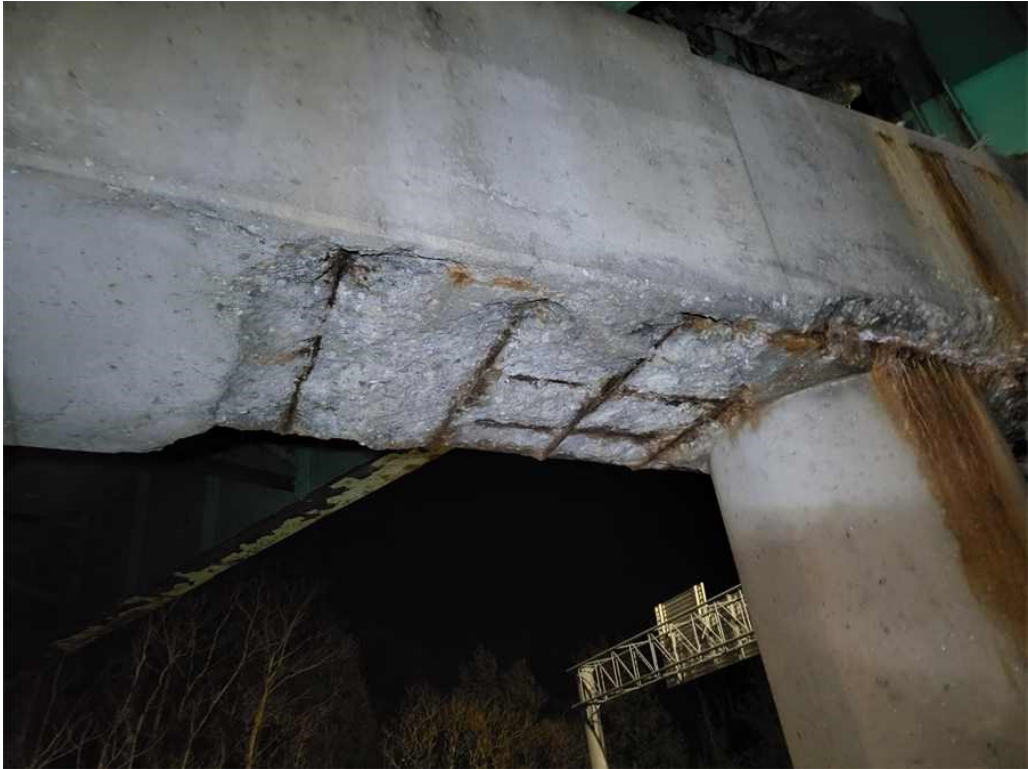
Photo 53: Pier cap, bottom face, between Columns 3 & 4: severe spalling adjacent to Column C4 with exposed rebar.
