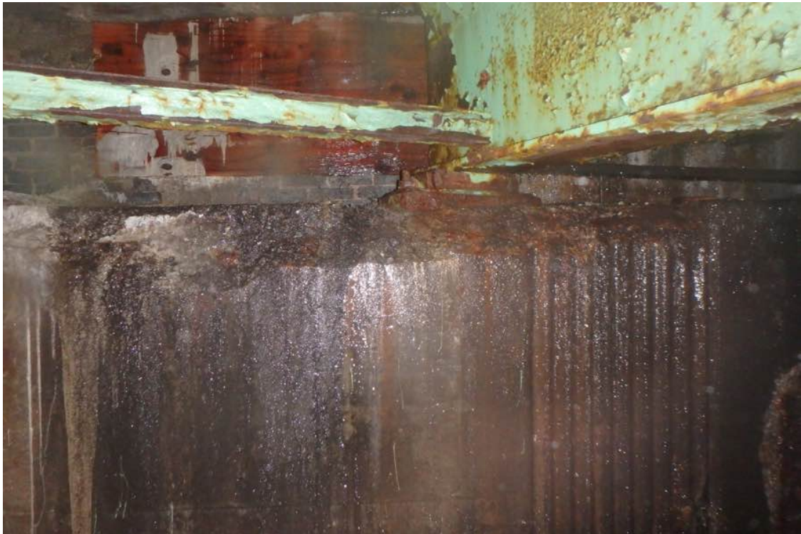
Photo 32: North breastwall, spalling along the top edge of Bays 1 & 2.
