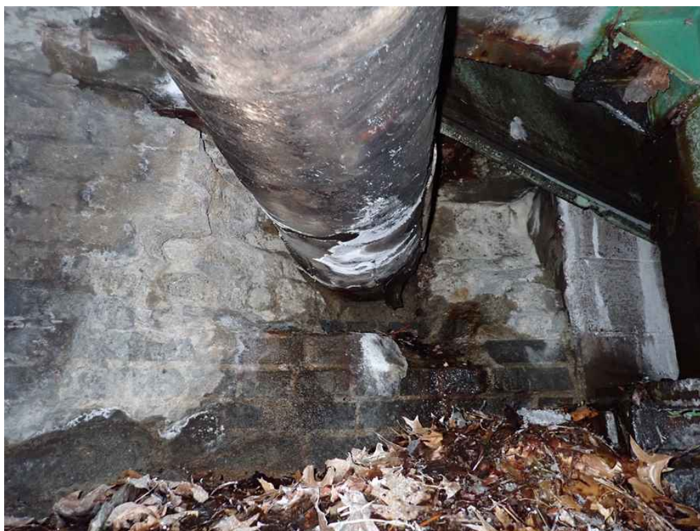
Photo 30: South Backwall in Bay 12 with deteriorated and missing bricks.
