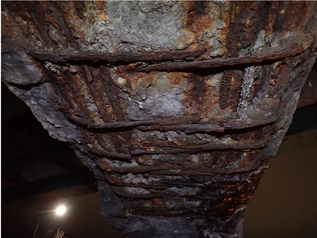
Photo 41: Pier cap underside between Columns 5 and 6 with 100% section loss to two stirrups.
