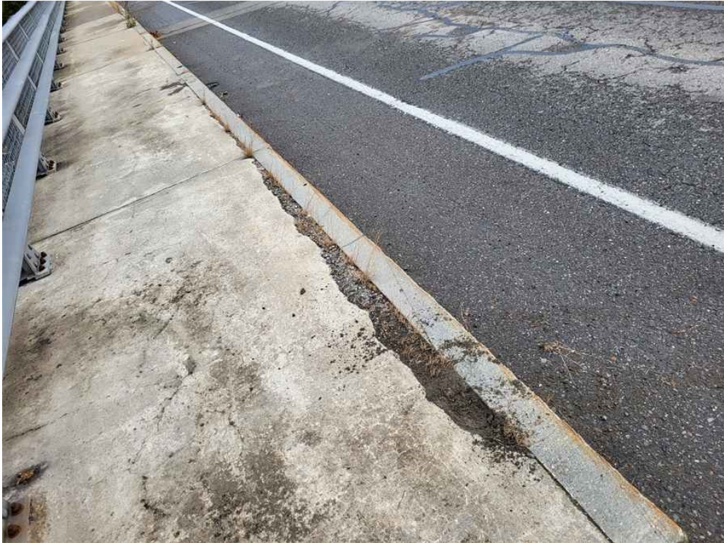
Photo 19: West curb, span 1, edge spalling behind the curb, up to 10' long x 6" wide x 1.5" deep. (Looking North).
