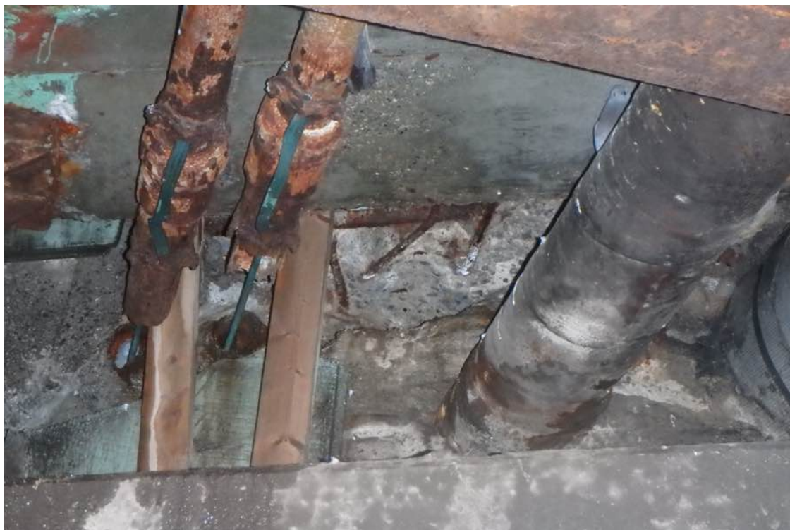
Photo 20: Bay 10 utility pipes rusted through at the north backwall. Note the spall in the backwall.
