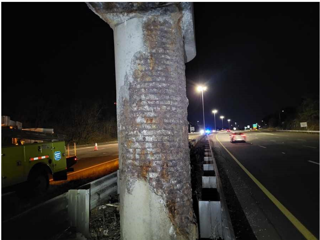
Photo 59: Column C1: severe spalling throughout the south and west face, full height x up to 4" deep, with exposed and rusted through rebar.
