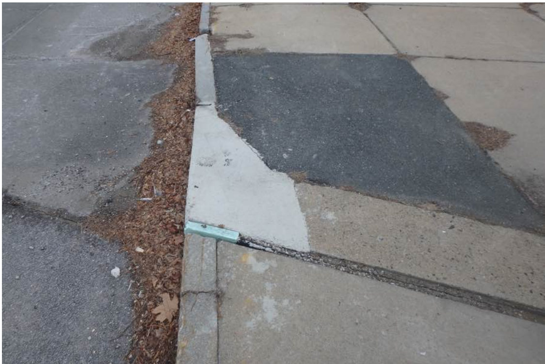
Photo 14: East curb, repaired section in the north approach corner.
