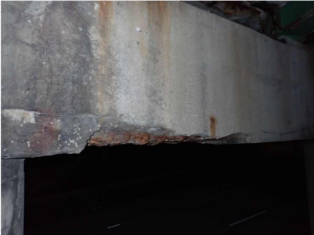
Photo 42: North face, between columns 5 and 6 with spall along the bottom.
