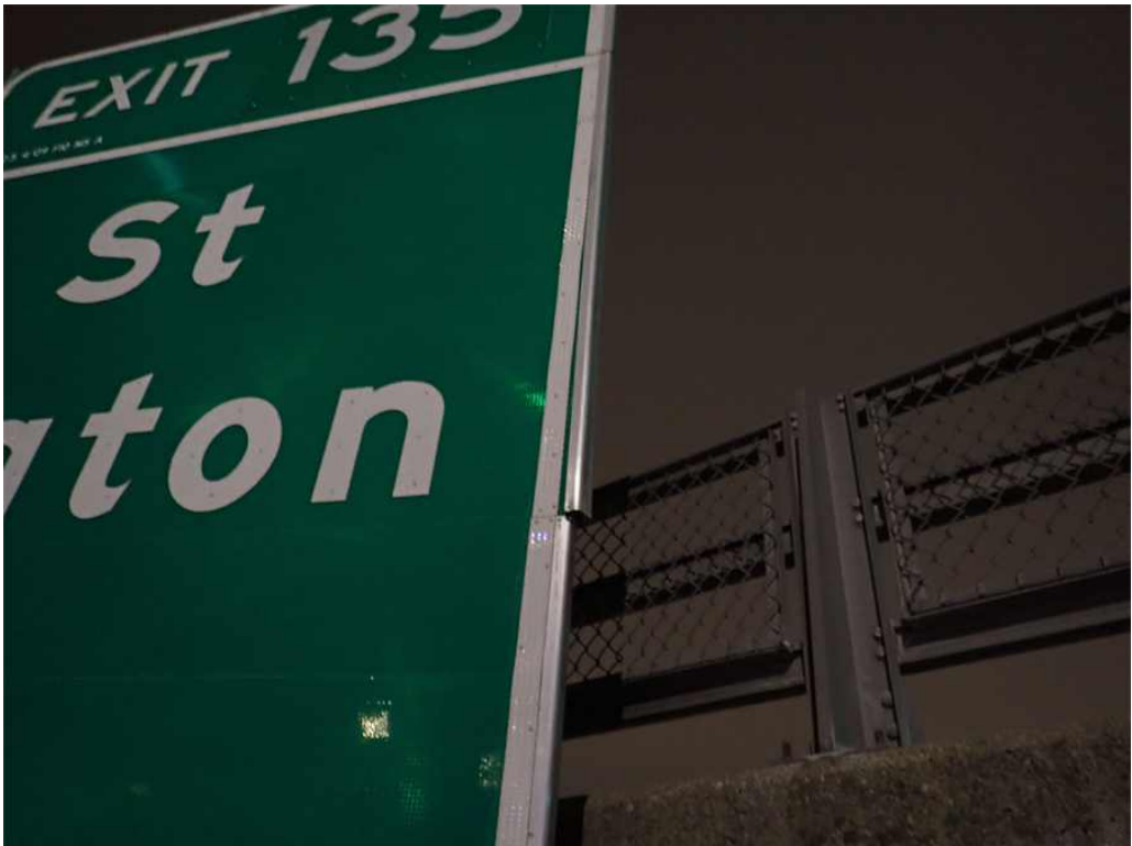
Photo 20: ST-2 eastbound overhead sign - Separation of the south edging near mid-height.
