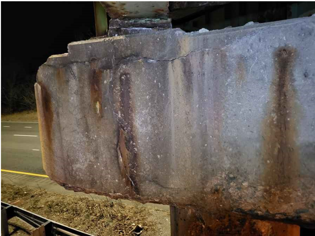
Photo 48: Pier cap south Face west end: 7' long x 1/4" wide horizontal crack at the top under girder G14 and a full height vertical hairline crack with rust staining and light efflorescence.
