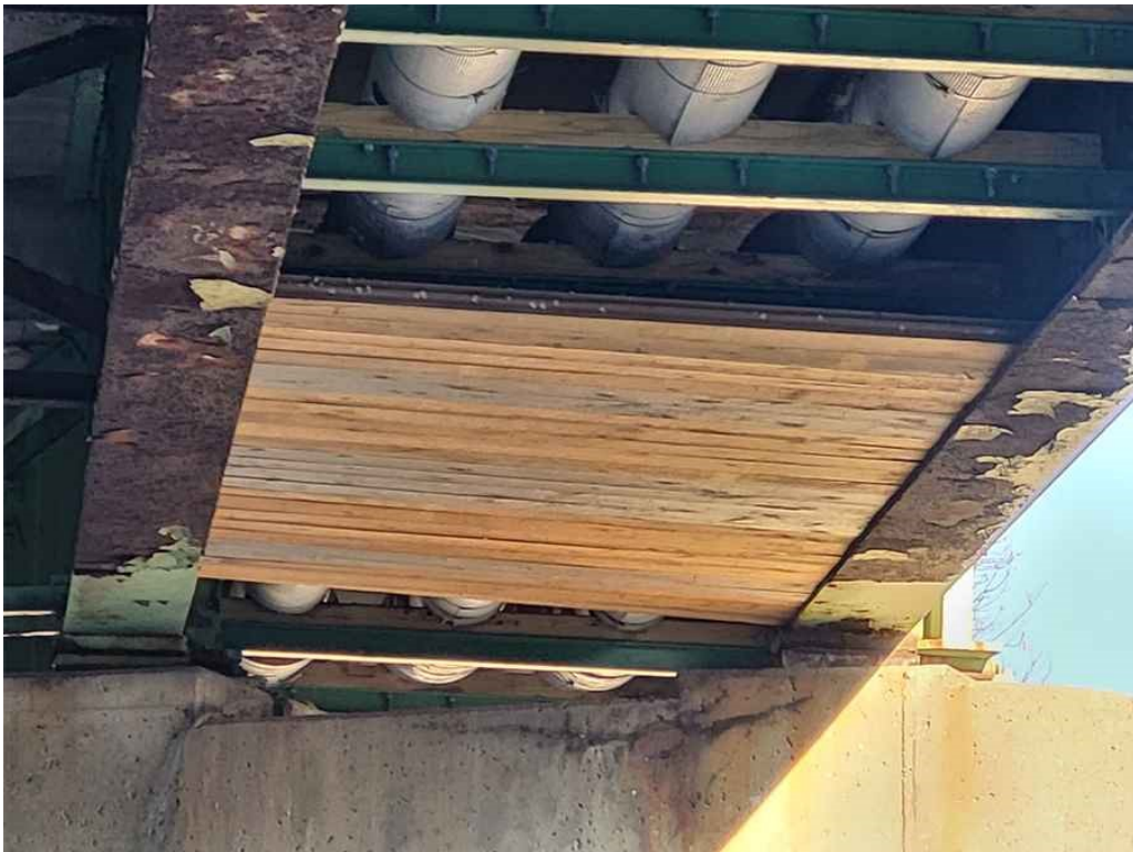
Photo 10: Deck, span 2, bay 7: timber shielding at the pier over the left travel lane.
