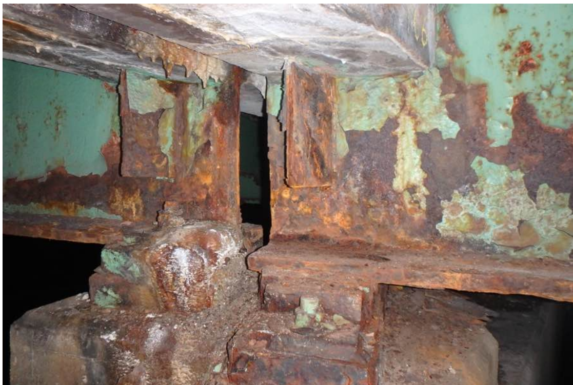
Photo 26: Typical rust and delamination throughout all beam ends at the pier joint.
