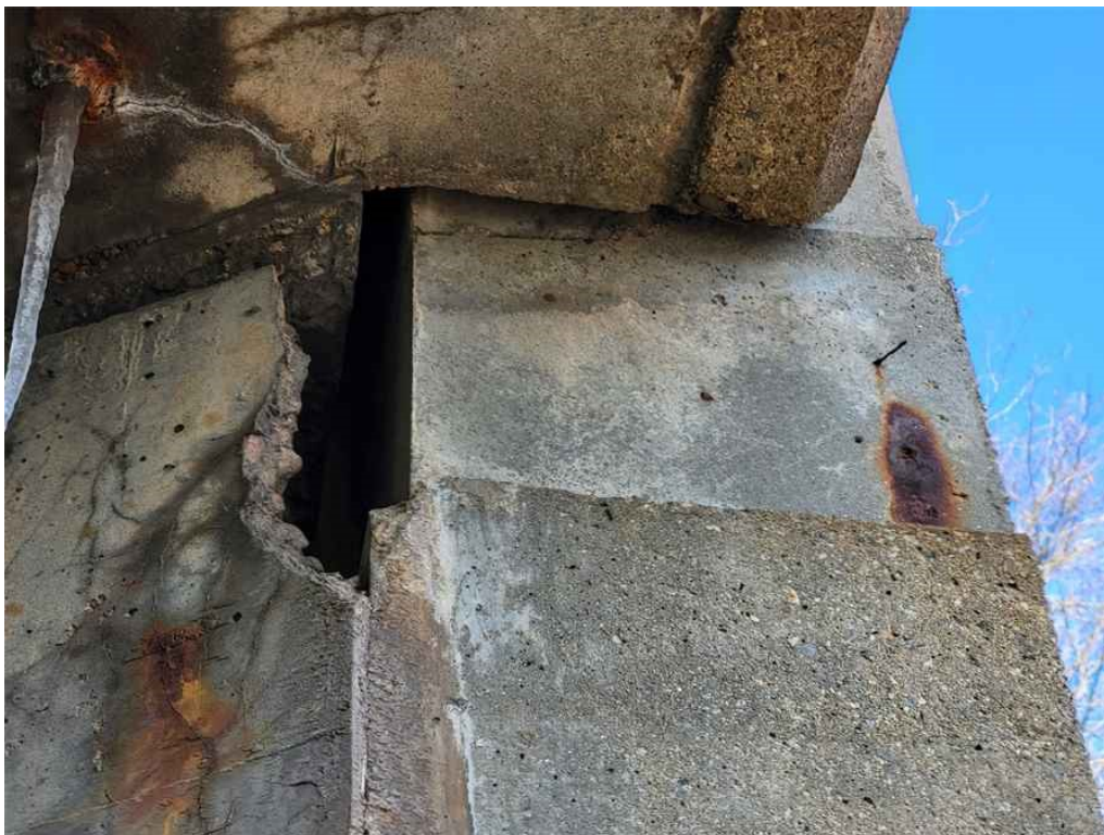
Photo 40: North Backwall, east end at the top, 1' high x 6" wide x up to 10" deep spall.
