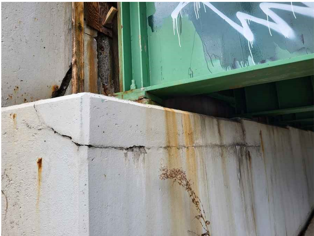
Photo 53: South breastwall, east corner: horizontal crack under bays 6, full bay length x up to 1/8" wide.
