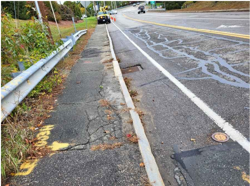
Photo 34: Northwest approach sidewalk: the asphalt portion exhibits heavy map cracking with several areas of depression. (Looking North).
