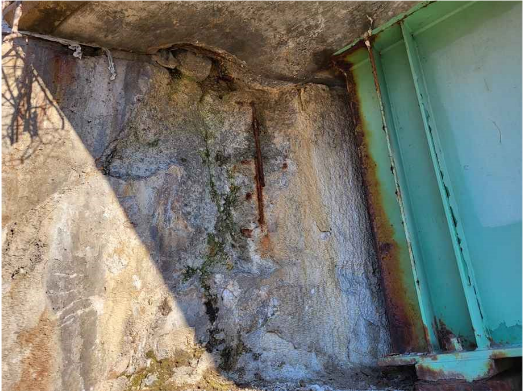
Photo 41: West end of the north backwall: full height x 3.5' wide x 8" deep spall with exposed rebar.
