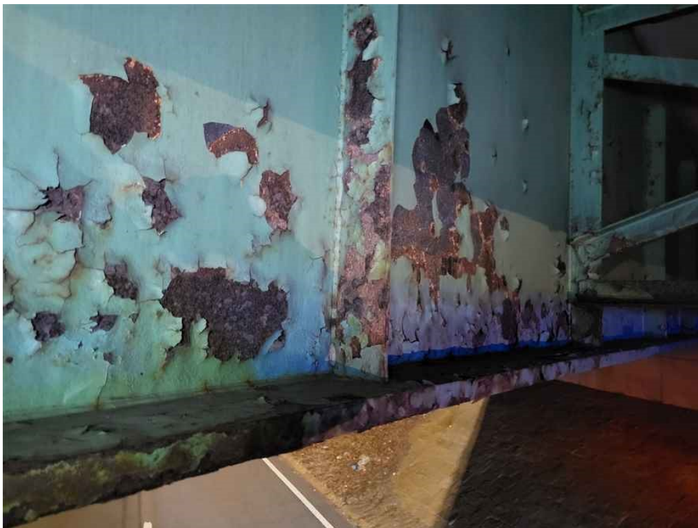
Photo 26: Steel girders: chalky peeling paint with moderate to heavy rusting. (Girder G5 shown, Looking Northwest).
