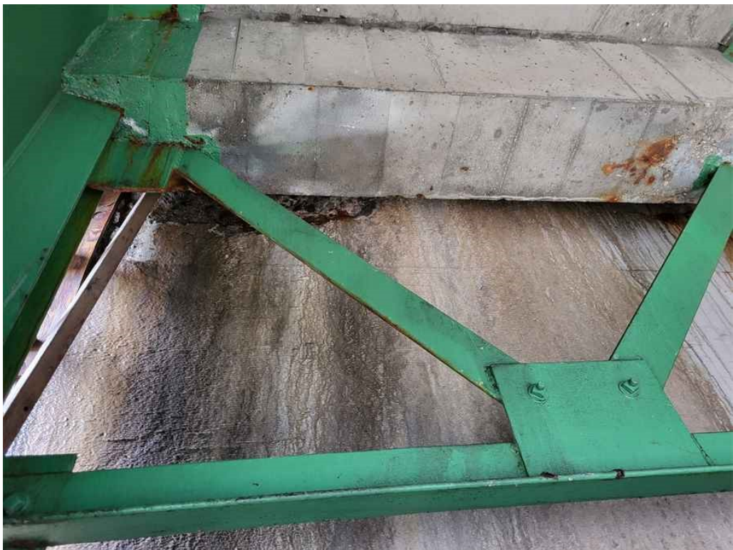
Photo 49: South backwall, bay 6: spall at the top, 2' wide x 1' high x 1.5" deep.
