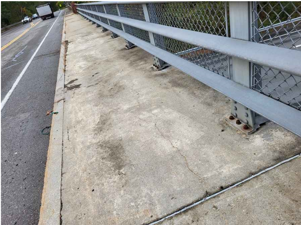
Photo 20: West curb: longitudinal hairline cracking that continues up to full span 2 length. (Looking South).
