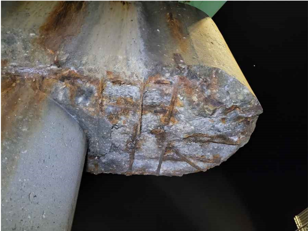
Photo 54: Pier cap, bottom face, west nose area: severe spalling with exposed and broken rebar.
