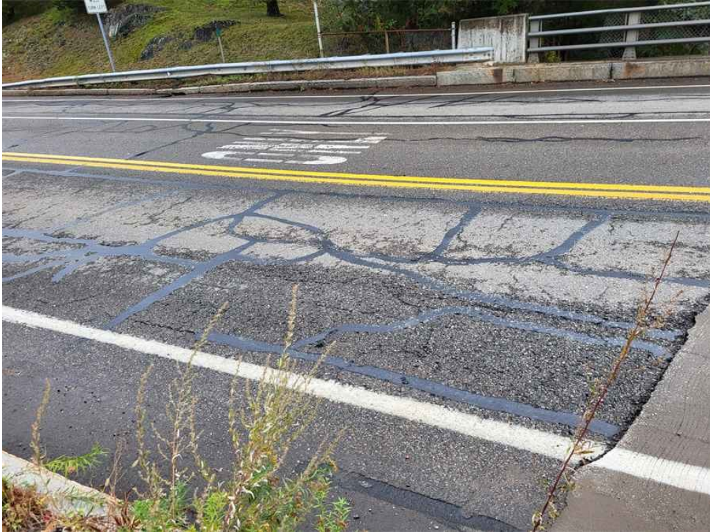
Photo 30: Approach roadways: several sealed and non-sealed longitudinal and transverse cracks throughout both travel lanes, up to 1/2" wide (North approach shown).
