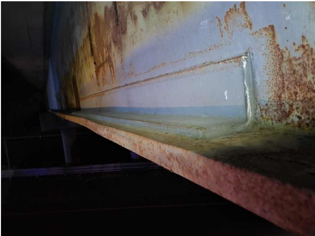
Photo 28: Girder 1, span 1: minor impact damage to the bottom flange and web at mid-span over the 2nd right lane. (Looking South).
