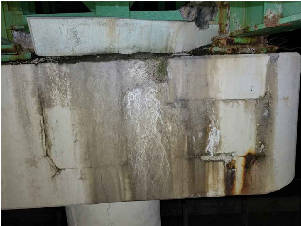
Photo 62: Pier cap, south face, bay 6, three spalls, rust staining and efflorescence, up to 9" diameter x 1.5" deep and several vertical and horizontal crack with active leakage.
