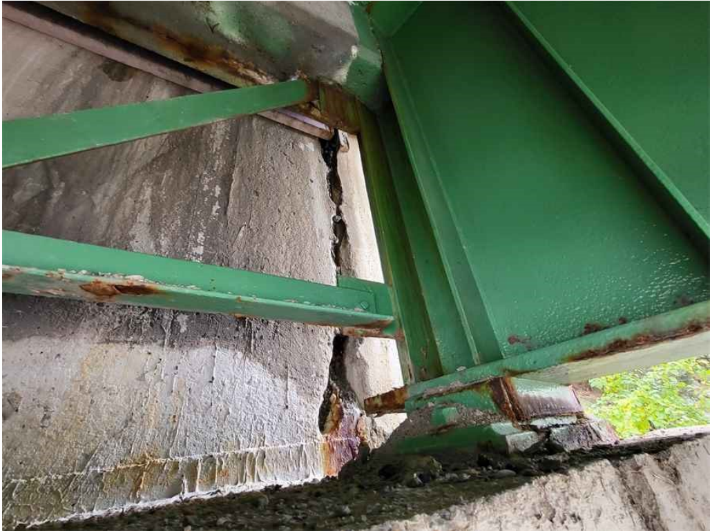
Photo 51: North backwall, behind beam 14: full height spall x 6" wide x 2" deep.
