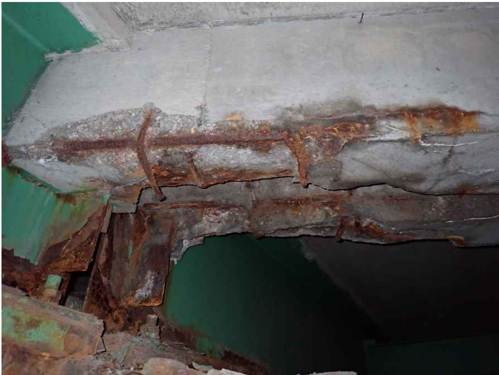
Photo 26: Typical spalling with exposed rebar to the concrete end diaphragms.
