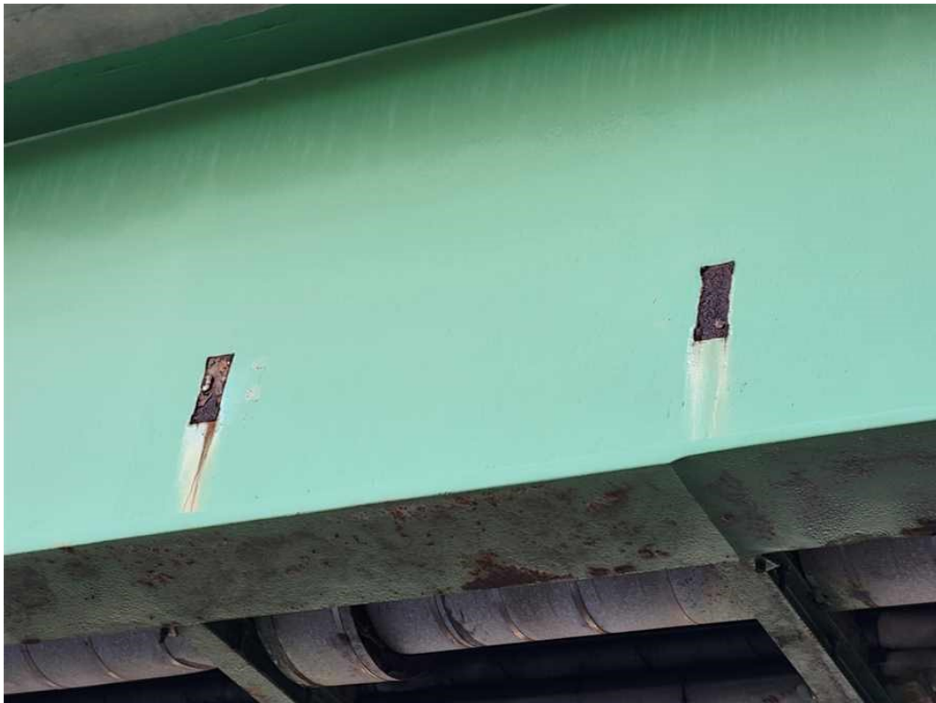
Photo 36: Beam 1, span 1, west face: two rusted areas of an old bracket that was previously removed.
