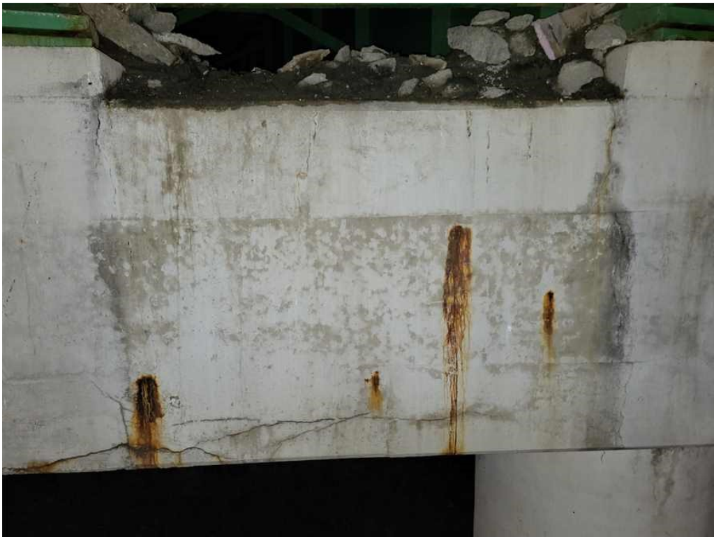
Photo 64: Pier cap, north face, bay 4, horizontal cracks at the bottom, up to full bay length x 1/8" wide, several spots of rust staining and full height x 1/8" wide vertical crack under beam 11.
