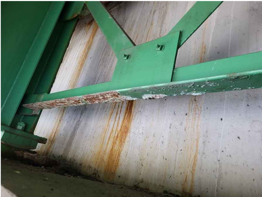
Photo 48: Bottom chord of the first cross frame at the south abutment (span 1, bay 5), light surface rust, paint peeling and light accumulation of efflorescence.
