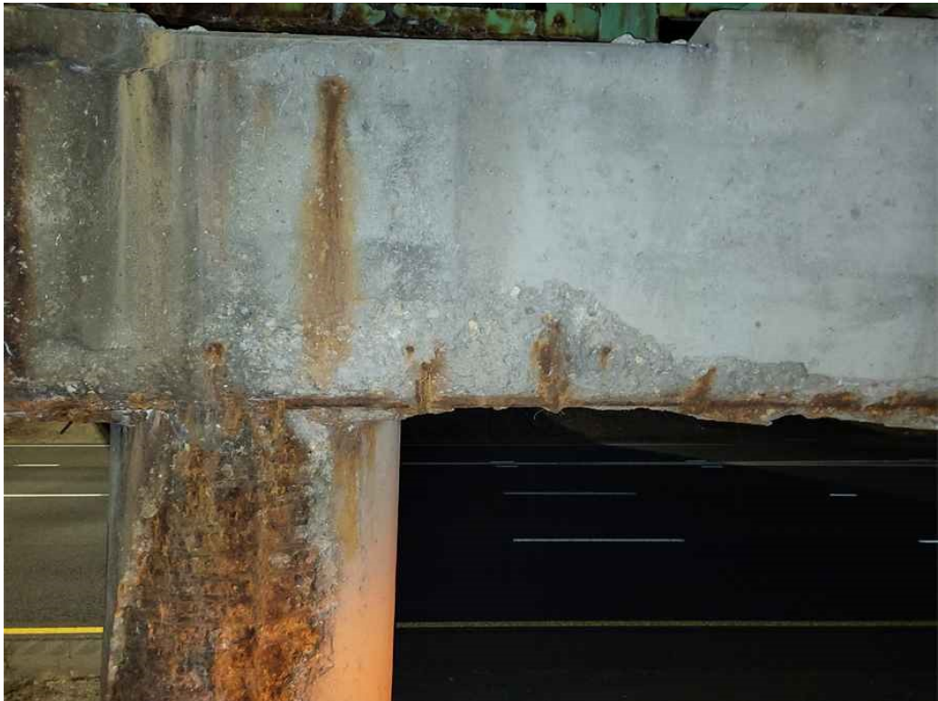
Photo 49: Pier cap, south face: starting between Columns 3 & 4 and ending at the west end, spalling along the bottom edge extending into the bottom face with exposed and rusted rebar.
