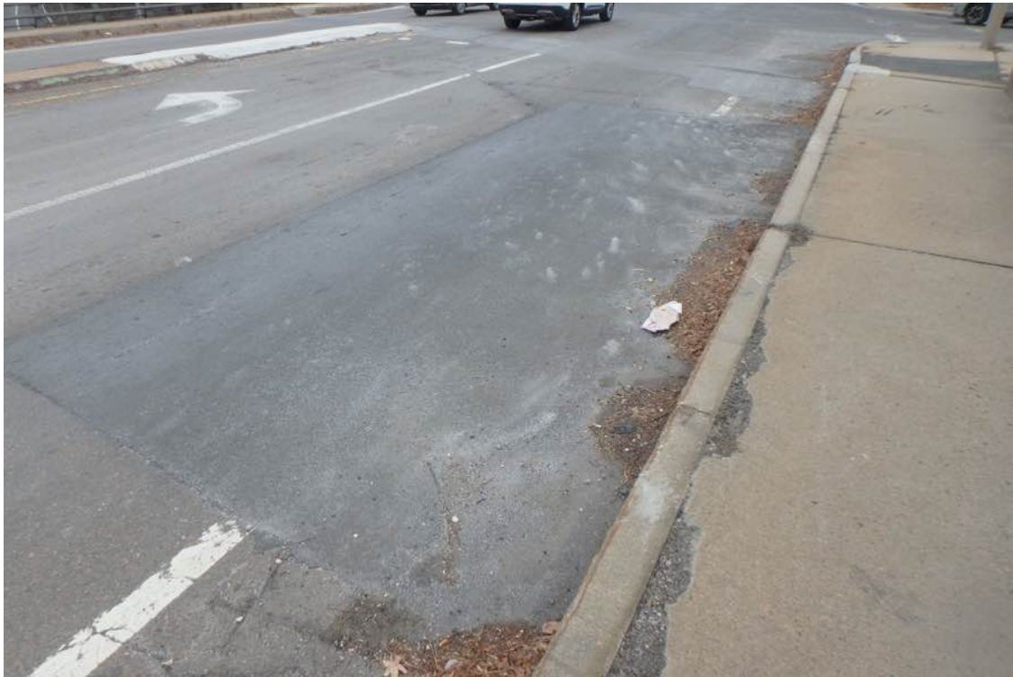
Photo 5: Northbound roadway, patch just south of the north abutment joint. Note the repaired nose to the median.
