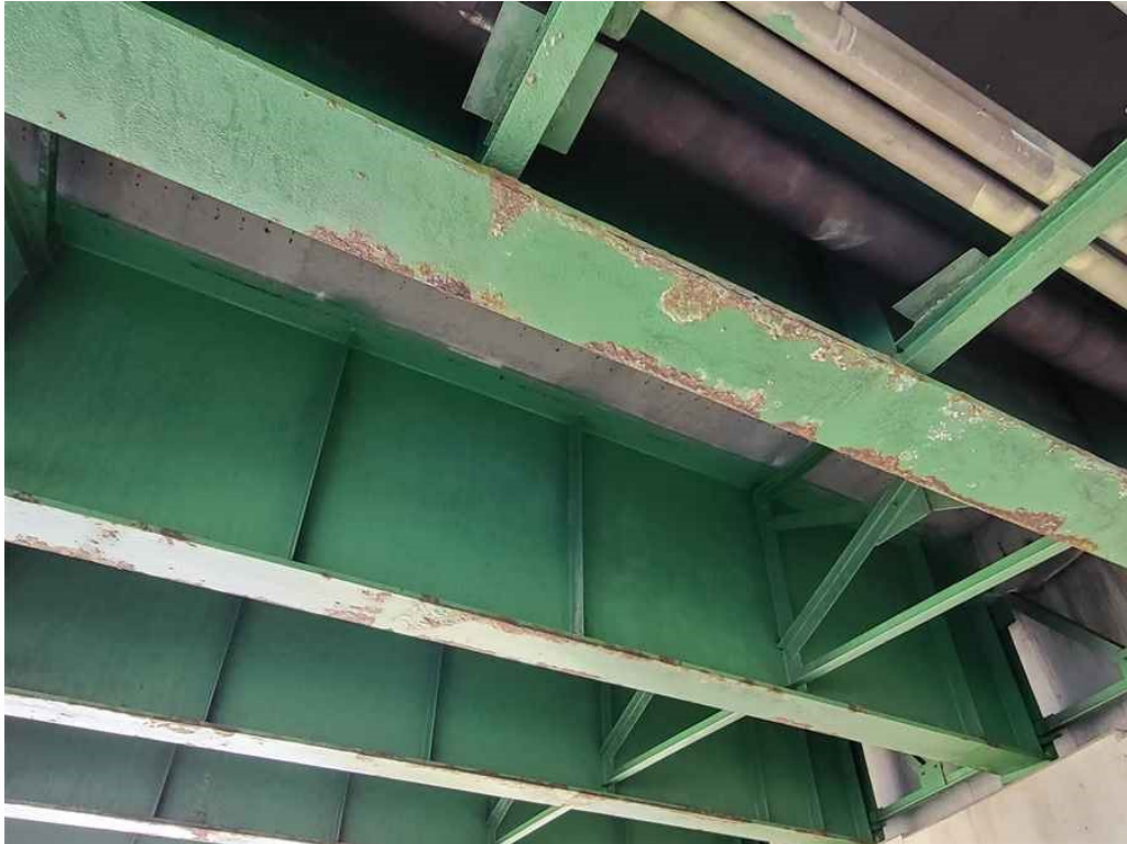
Photo 35: Beams: typical random areas of minor rusting to the bottom flange. (Beams 2 - 4, span 1 near south abutment shown).
