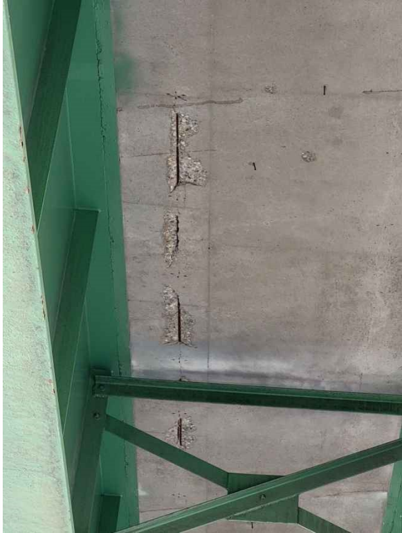
Photo 11: Deck, span 2, bay 3 near mid-span: several spalls running parallel to Beam 11 with exposed rebar.
