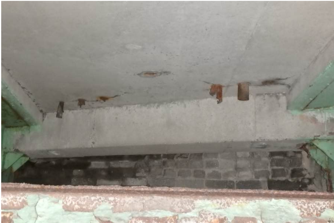
Photo 17: Span 1, Bay 1 weep-holes with no PVCs extending below the bottom flanges.
