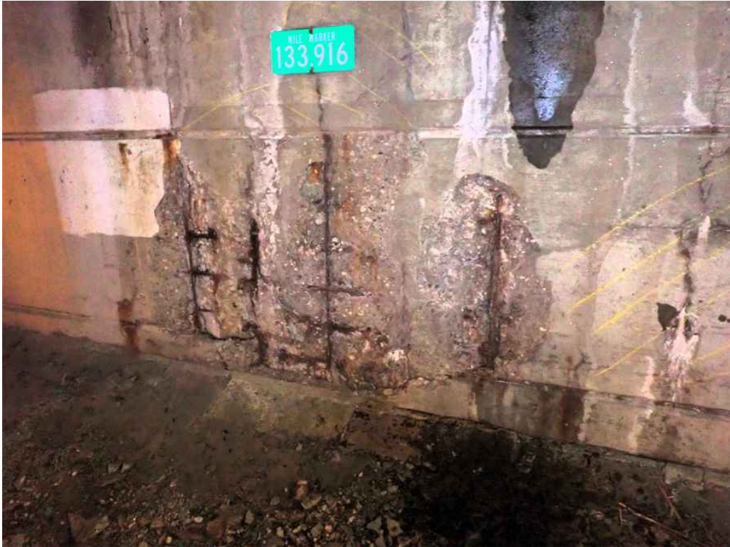
Photo 35: North Breastwall under Bays 11 and 12 with spalling, exposed rebar, and delaminations.
