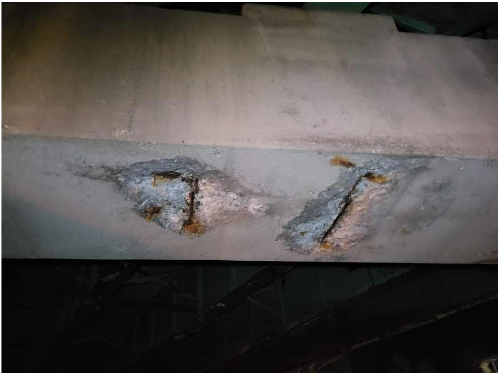
Photo 52: Pier cap, bottom face, between Columns 2 & 3: two spalls with exposed rebar.
