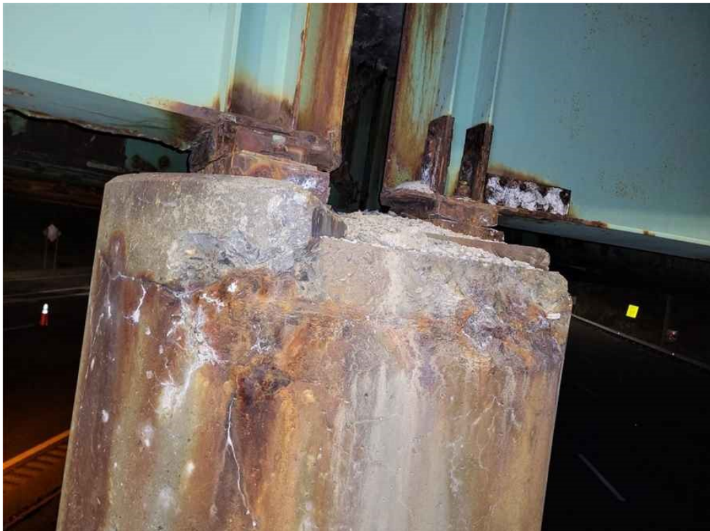
Photo 58: Pier cap, west nose: spalling along the top edge with exposed and rusted through rebar.
