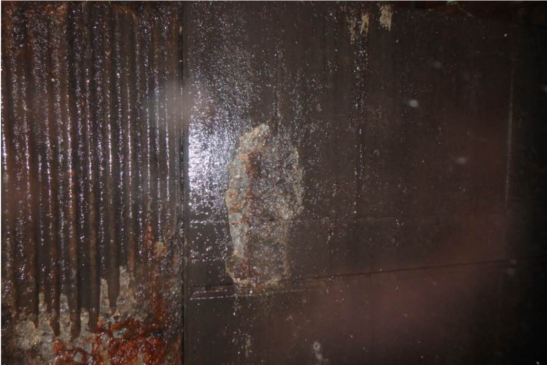
Photo 34: North breastwall, Bay 2 spalling near the top.
