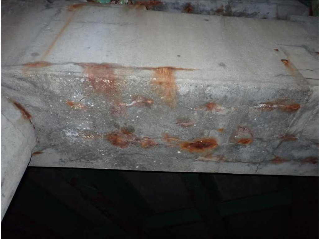
Photo 37: Pier Cap underside between columns 2 and 3 with cracking, rust staining, and delamination.
