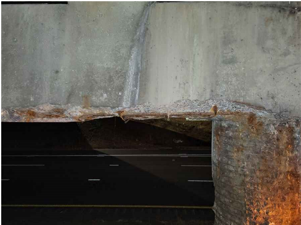
Photo 50: Pier cap, south face, between C1 & C2: spalling along the bottom edge extending into the bottom face with exposed and rusted through rebar.
