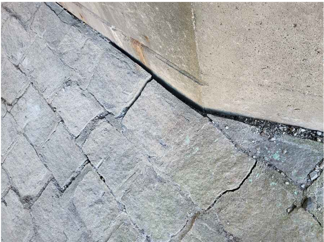
Photo 46: South stone slope protection: 2.5" wide separation from the abutment breastwall. (West end shown).
