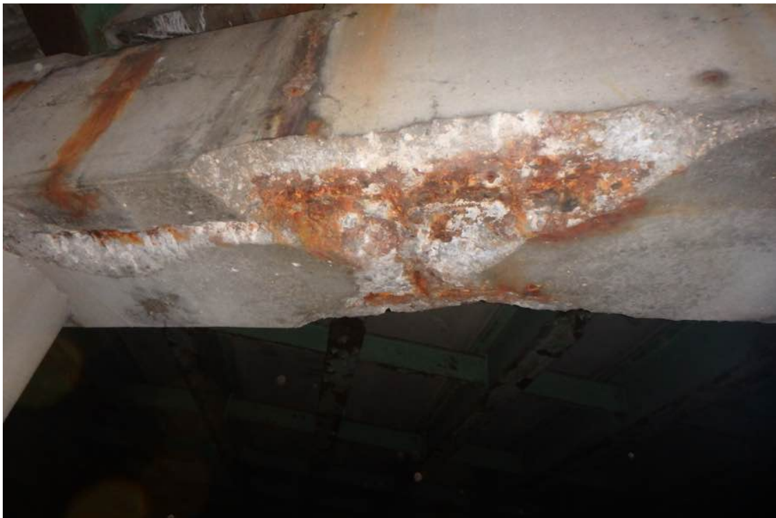
Photo 44: Pier cap, spall between Columns 3 & 4.
