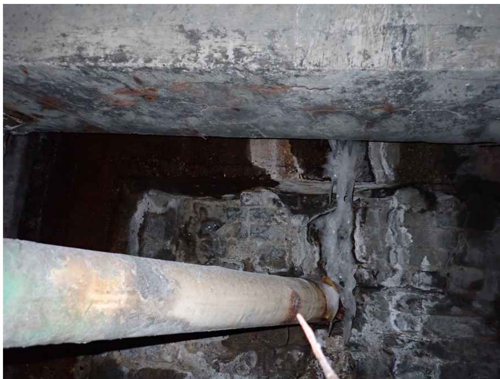
Photo 29: South Backwall in Bay 1 with deteriorated and missing bricks.
