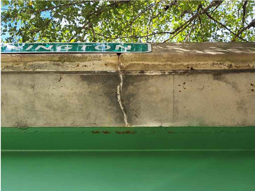
Photo 5: Deck overhangs: Typical random full width hairline cracks, some with light efflorescence.
