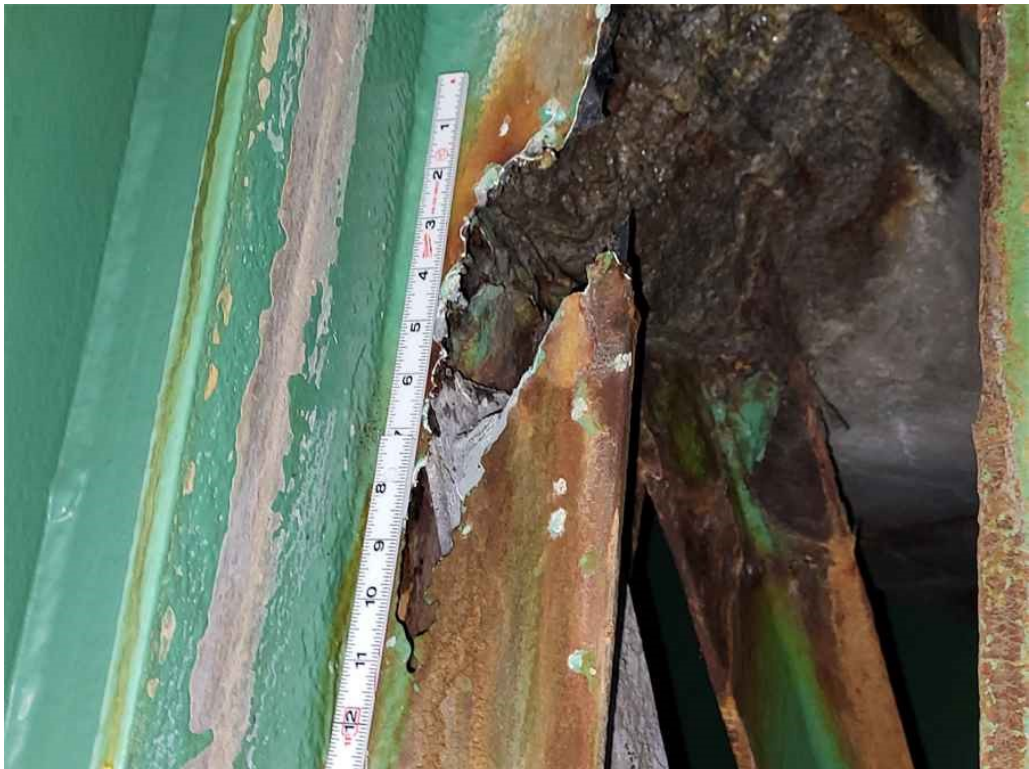
Photo 38: Beam 7: areas of 100% section loss at the north end of the web beyond the bearings measuring 10" high x 3" wide near mid-height.
