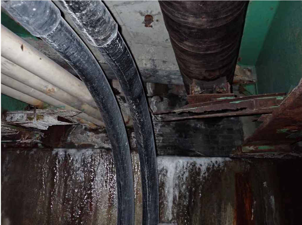
Photo 9: 100% section loss to the south utility support bracket in Bay 1 of Span 1.
