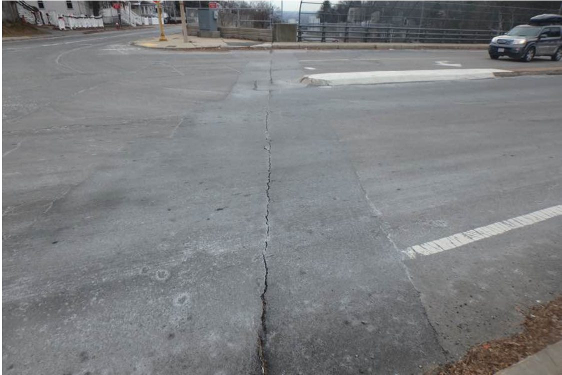
Photo 3: North abutment joint. Note the full length crack in the joint and repaired nose to the median.
