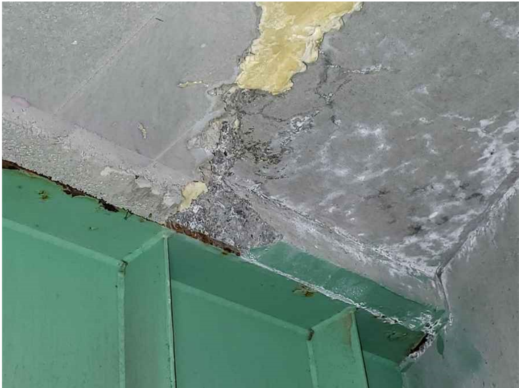
Photo 11: Deck, span 2, bay 11: haunch spall near girder G13 , up to 1' long x 3" deep x 3" wide and adjacent hairline map cracking with light efflorescence.
