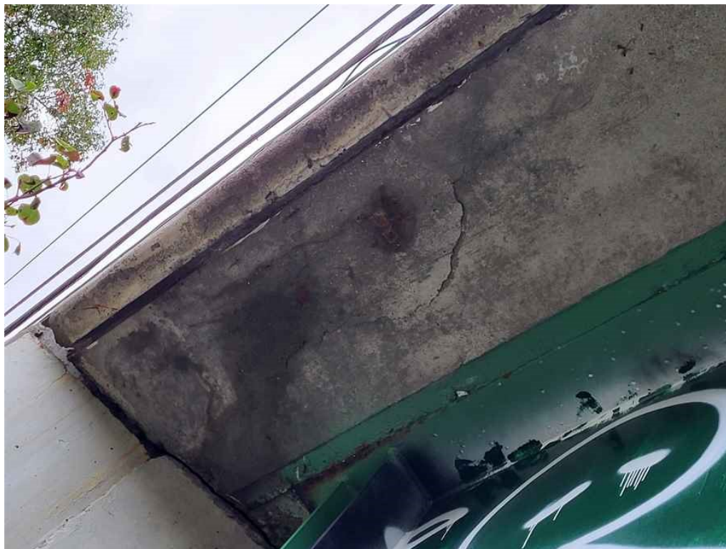
Photo 10: Deck, west overhang at north abutment: up to 2.5' long x 1.5' wide area of delamination.
