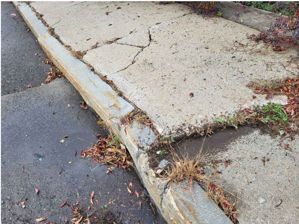
Photo 32: Southwest approach sidewalk is heaved, up to 2" along with diagonal and longitudinal corner cracks, up to 1/2" wide. (Looking South).
