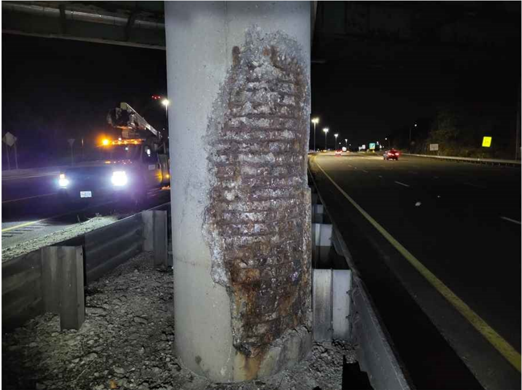
Photo 61: Column C3: moderate spalling throughout the bottom half of the southwest face, 7' high x 4' wide x 4" deep, with exposed rebar.
