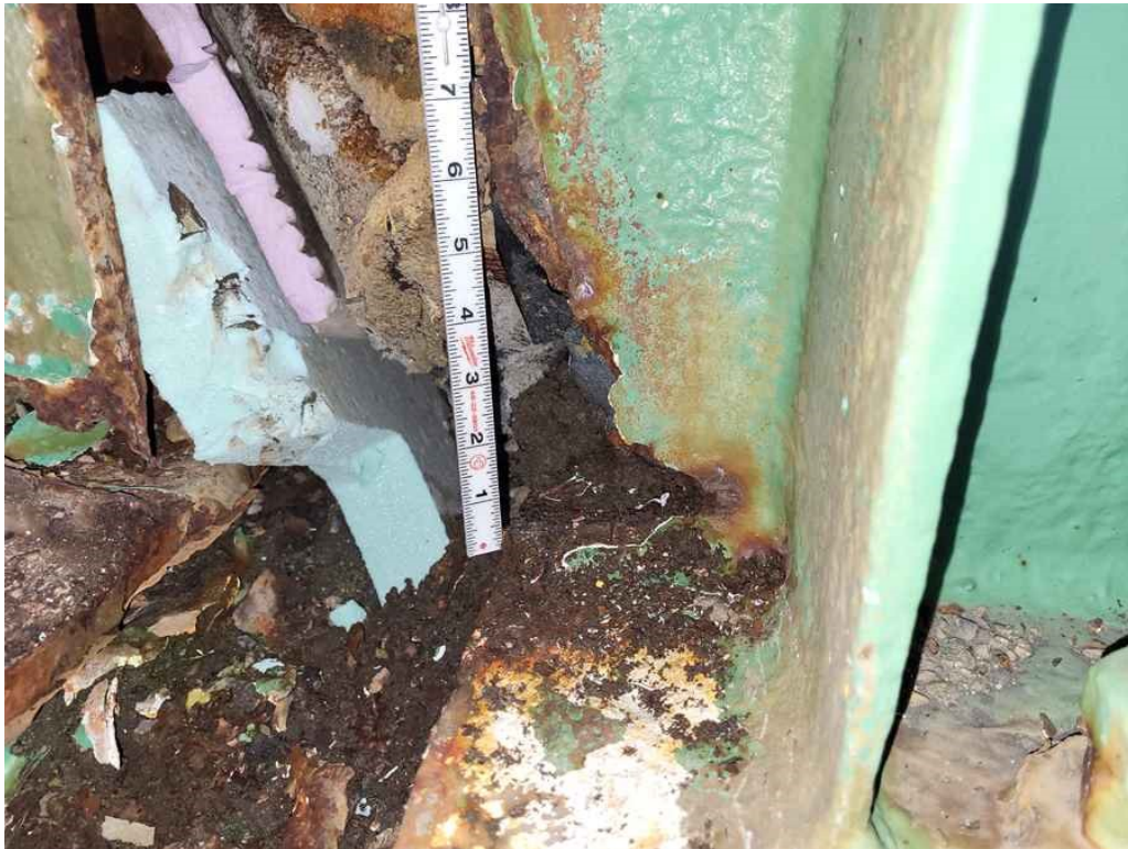
Photo 41: Beam 14 in span 2: areas of 100% section loss at the south end of the web beyond the bearings measuring 5" high x 3" wide at the bottom.
