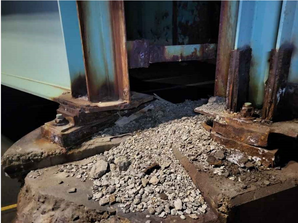
Photo 37: Bearings at the pier: moderate rusting and debris behind the bearings. (Bearings of beams G7 and G14 shown).
