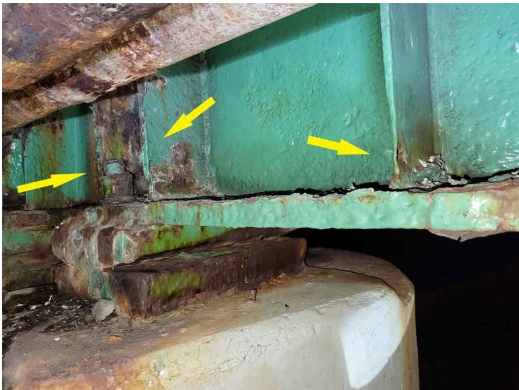
Photo 42: Beam 8: the southern most 3 vertical stiffeners on the east side of the web are knifed down significantly adjacent to the bottom flange. Also note the moderate rust to the bearing.
