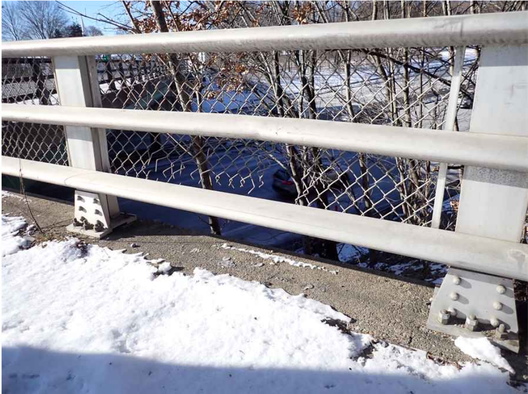
Photo 7: Minor damage to the west rail at the north end.
