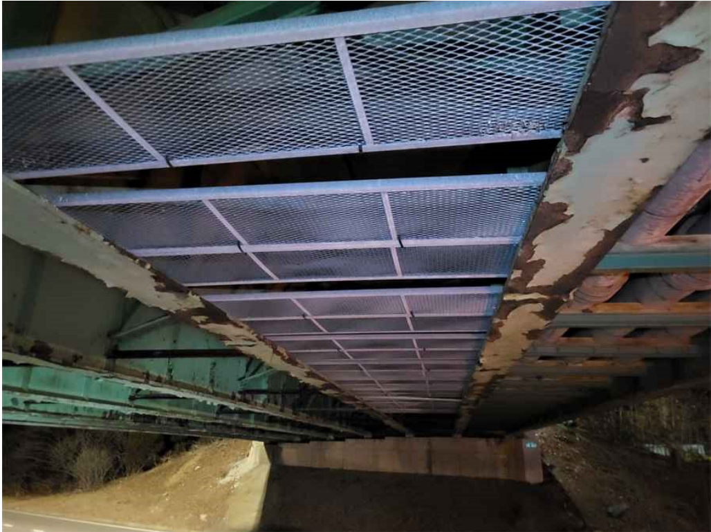
Photo 7: Deck, span 1, bay 2: metal screening between diaphragms 3 - 6.
