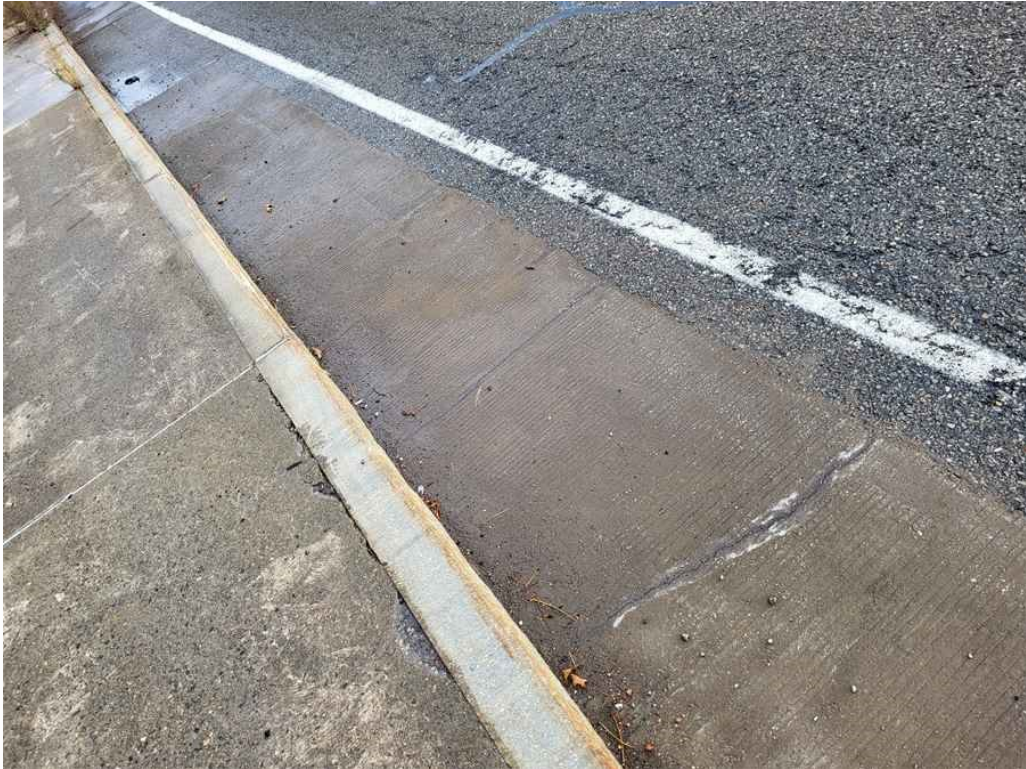
Photo 3: Wearing surface: typical full repair width transverse hairline cracks adjacent to the west curb.
