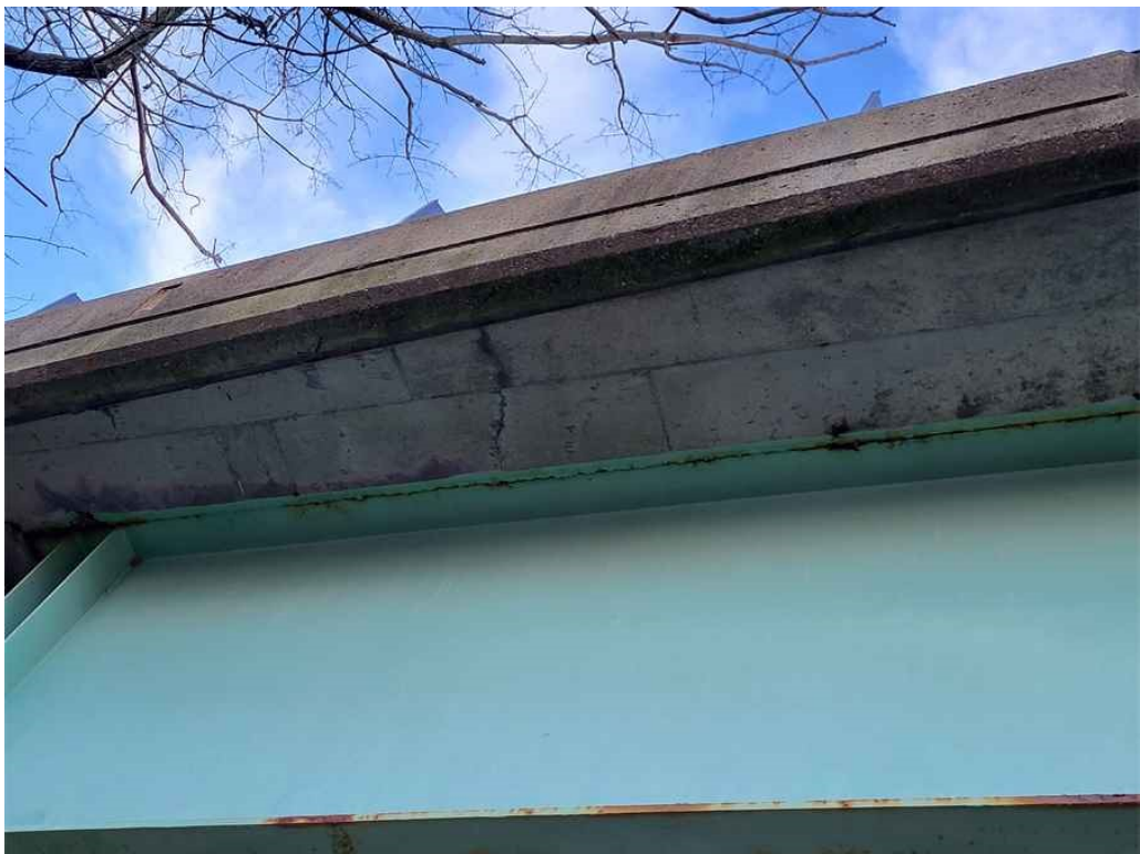
Photo 4: Typical hairline transverse cracks with light efflorescence throughout the deck overhangs. (Span 2, east overhang shown).
