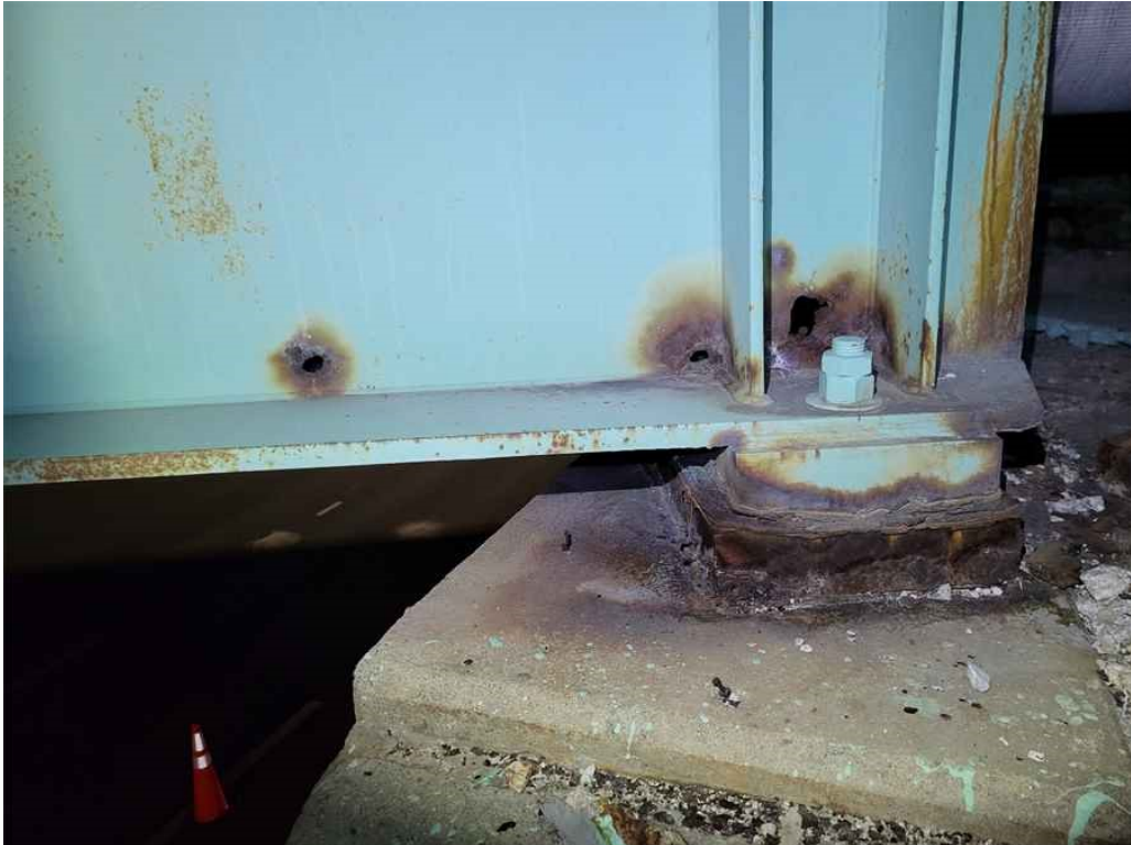
Photo 33: Girder 8, span 2: web with heavy rusting, 1" W x 2" H hole above the bearing, 1" Diam hole 2.75' from the end and 1" Diam hole just south of the web stiffener at the bearing. (East face shown).
