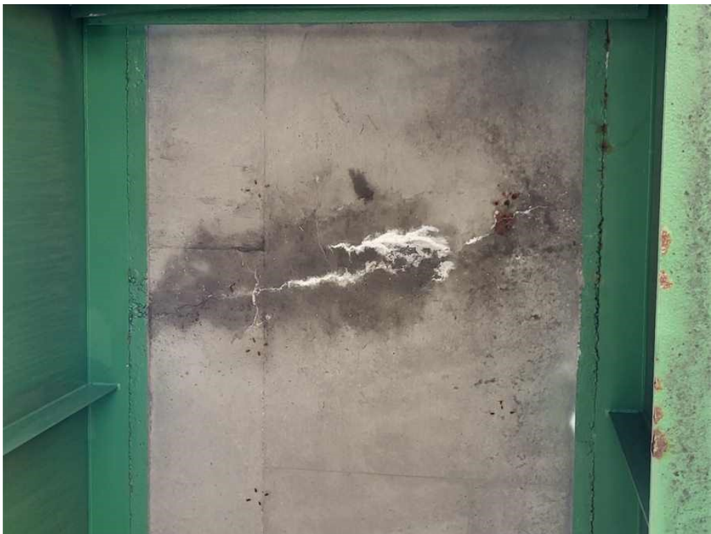
Photo 15: Deck, span 2, Bay 6: several random full bay width transverse hairline cracks with light efflorescence and dampness.
