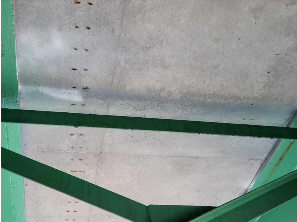
Photo 7: Deck, span 1, bays 2, 3, 5, 6: typical full bay width hairline crack over the second cross frame. (Bay 3 shown).
