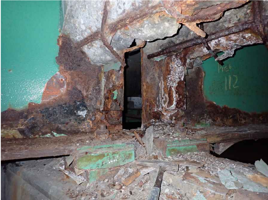
Photo 23: Beams 112 and 212 at the pier, west face, with rusting and section loss.
