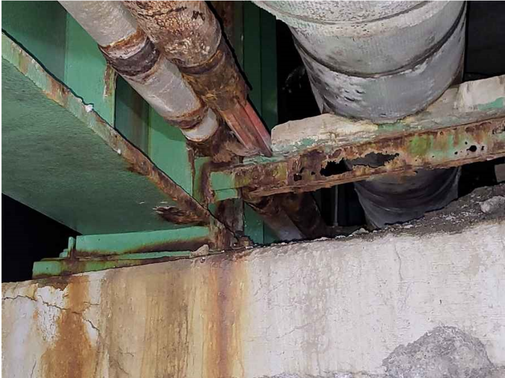
Photo 25: Bay 1, utility support bracket at the pier with severe rust and several areas of 100% section loss throughout. Also note the 100% section loss of the conduit pipes.
