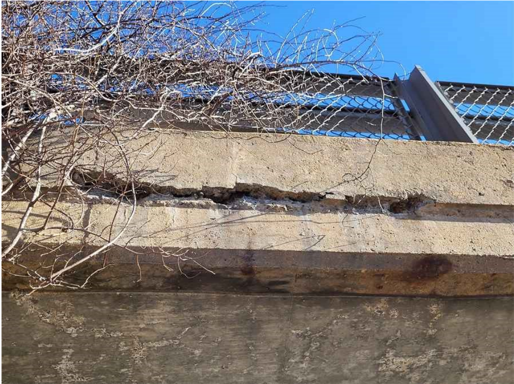
Photo 15: west fascia of the safetywalk: spalling, 4' long x 4" high x up to 3" deep near the north abutment and scattered areas of hairline map cracking.
