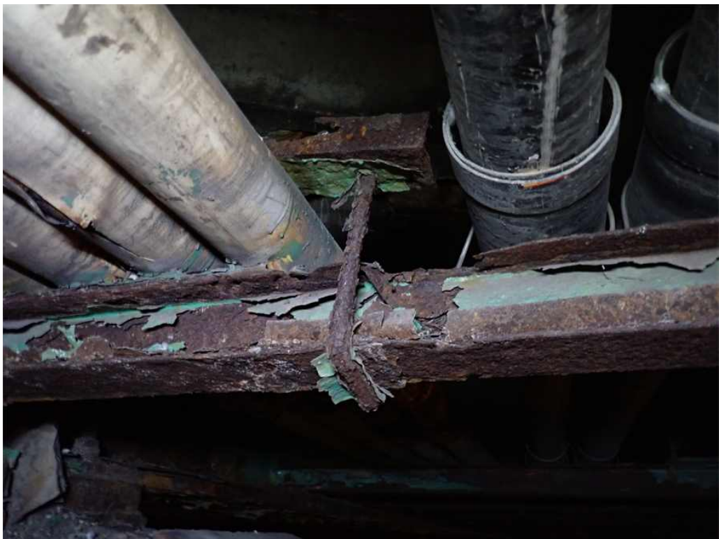
Photo 11: Severe laminar rust and section loss to the southern-most utility support in Bay 1 of Span 2 at the pier.
