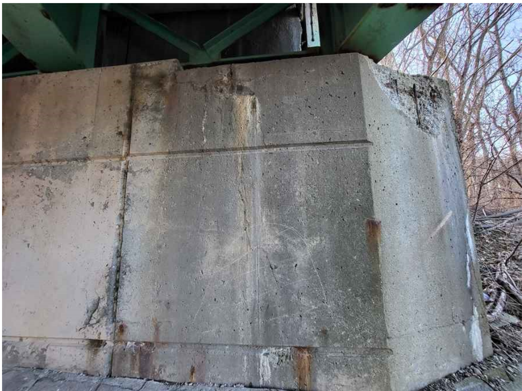
Photo 44: West end of south breastwall: spalls with exposed rebar, horizontal and vertical cracks with efflorescence and adjacent delamination area.
