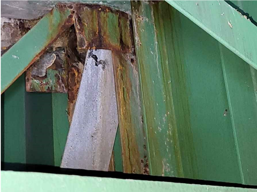
Photo 47: Connection plates of the cross frames over the pier in both spans: typical minor/moderate surface rust due to leakage from the joint above.
