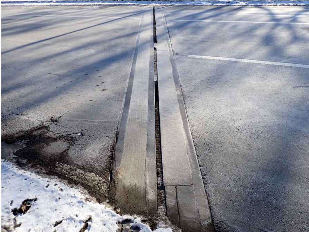
Photo 13: South abutment joint in the southbound lanes with displace filler martial.
