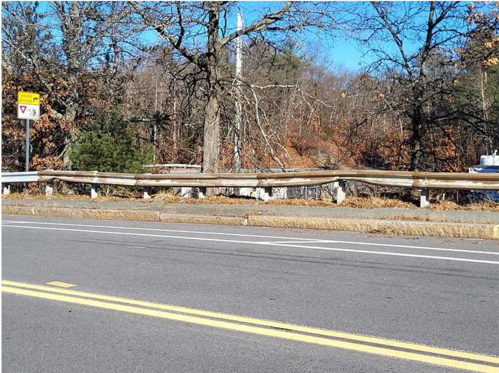
Photo 64: moderate collision damage at the northeast approach guardrail.
