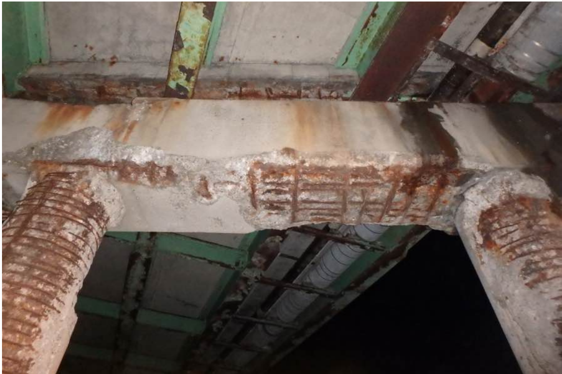
Photo 46: Pier cap, spall between Columns 5 & 6.
