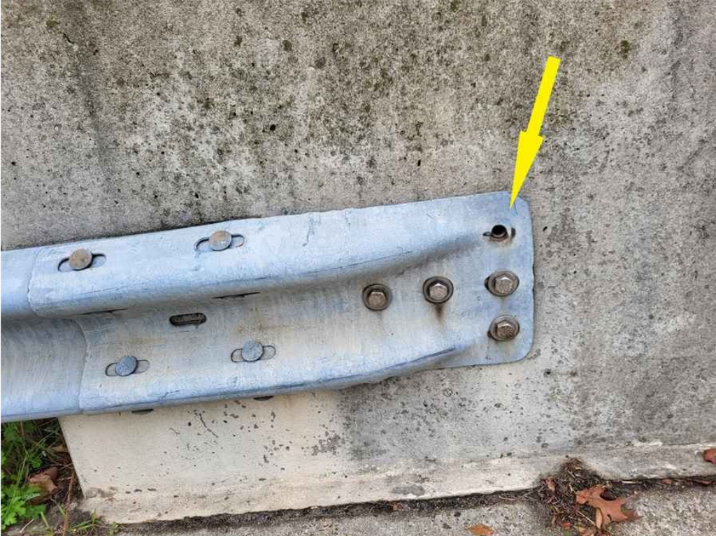
Photo 68: Southwest transitions is missing one bolt.
