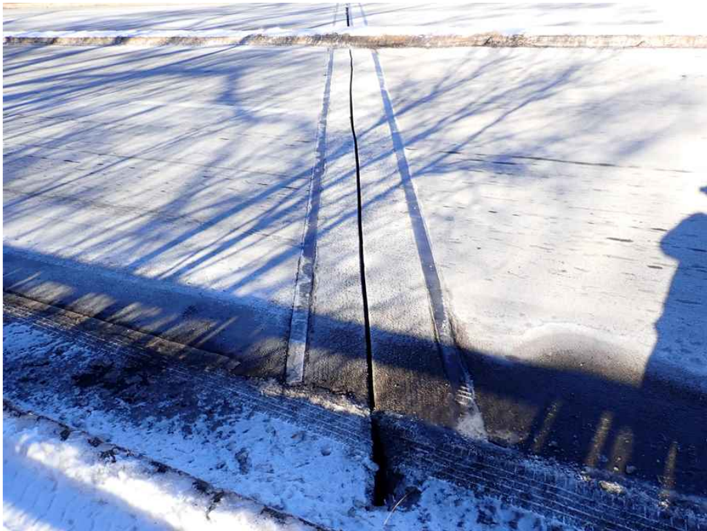
Photo 14: South Abutment joint in the northbound lanes.
