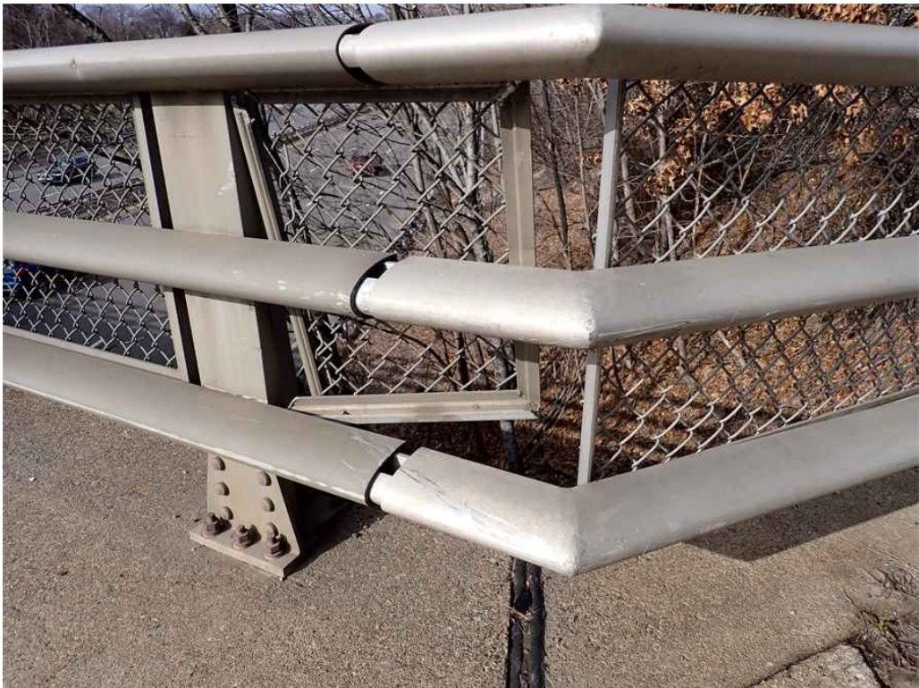
Photo 8: Minor damage to the west rail near the north end.
