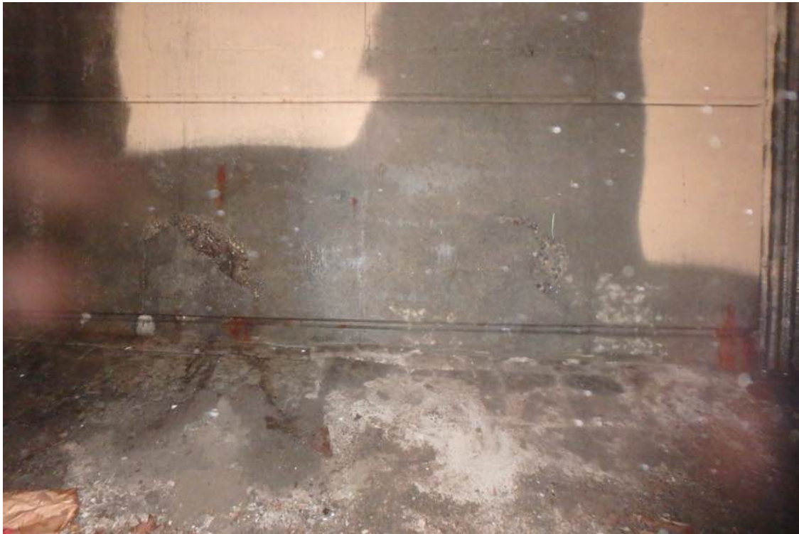
Photo 35: North breastwall, below Beams 204 & 205, spalling.
