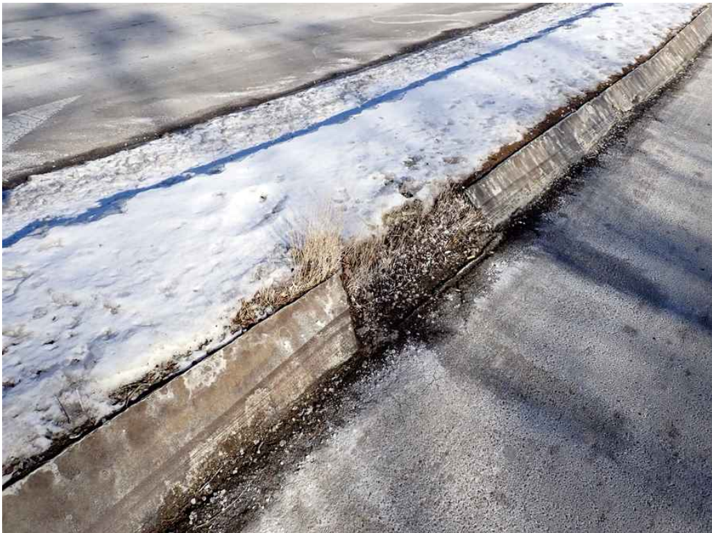
Photo 4: Median in Span 1 with missing curb section near the south end.
