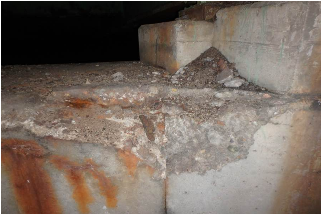
Photo 47: Pier cap, spall between Beams 205 & 206.
