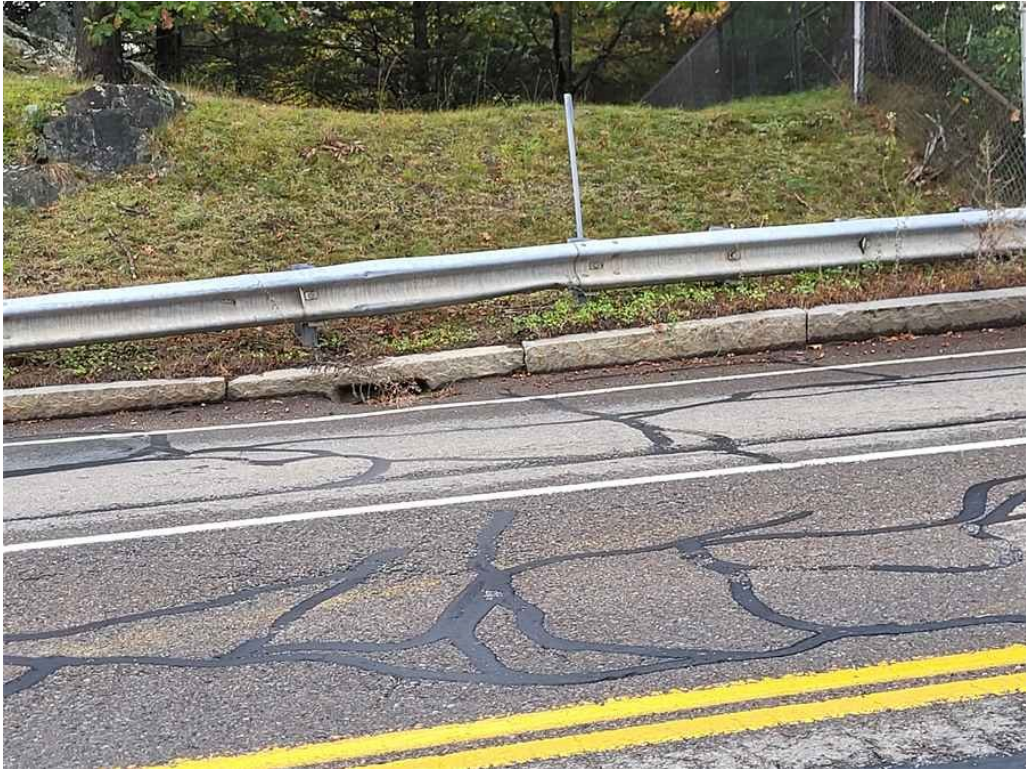
Photo 69: Northeast approach guard rail with minor impact damage.
