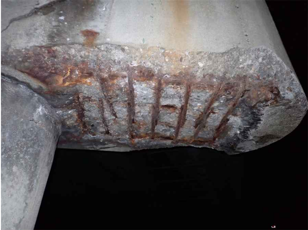
Photo 44: Pier cap underside at the east end with spall and exposed rebar.
