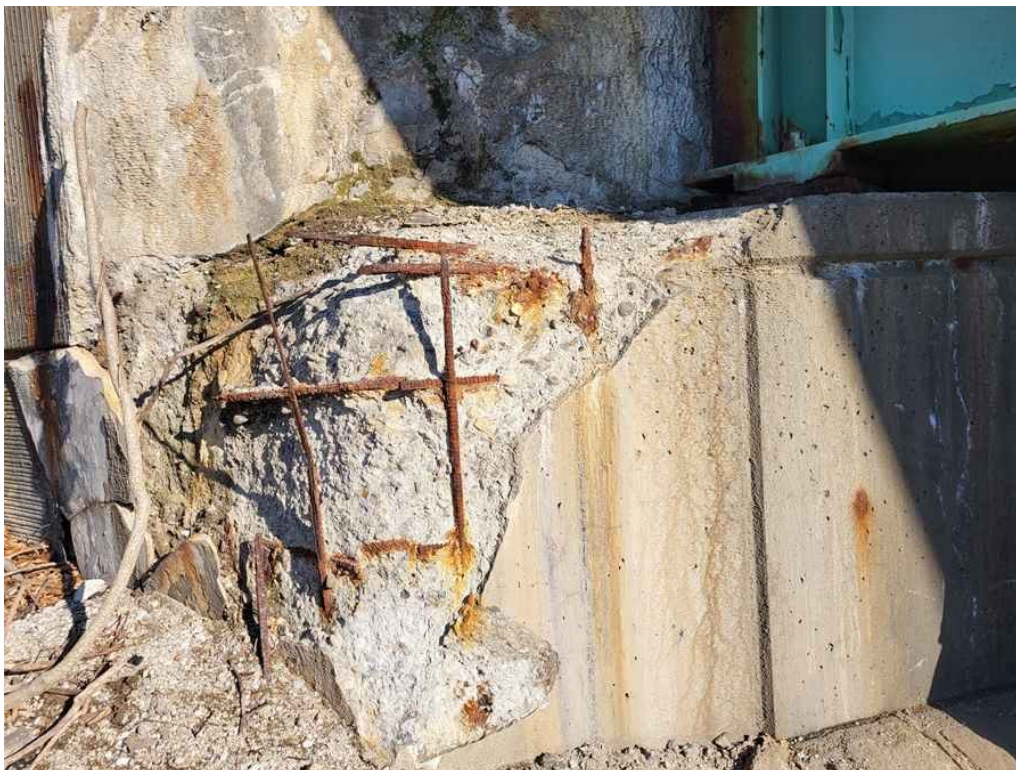
Photo 39: West end of the north bridge seat and breastwall: severe scaling/spalling with exposed, de-bonded and rusted rebar, full width, extending to Girder 7.
