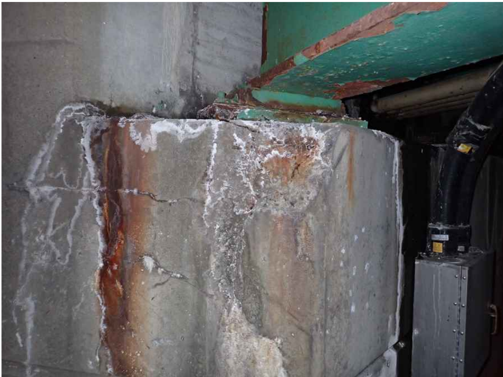
Photo 34: North Breastwall at the west end with spall and exposed rusted rebar.
