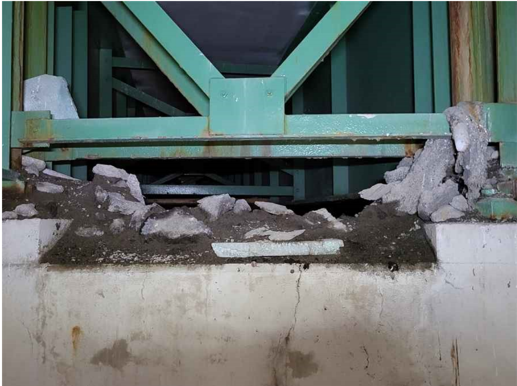
Photo 58: Pier cap, moderate debris and active leakage throughout the top of the pier cap. (Bay 4, south face shown).
