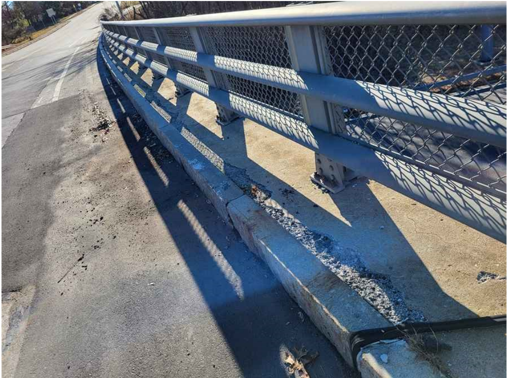
Photo 14: West safetywalk: large areas of severe scaling/spalling behind the granite curb up to 6" wide. (Span 2, Looking South).
