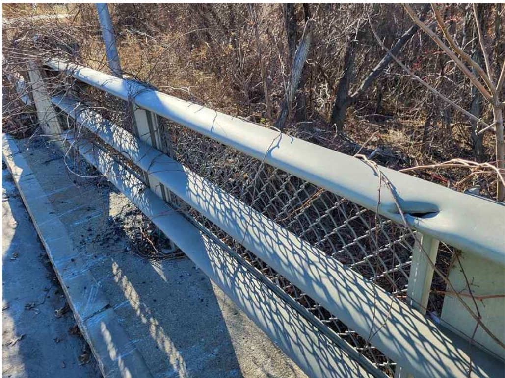
Photo 18: Bridge railing: small dent/tear at the top rail in several locations. (Southwest corner shown).
