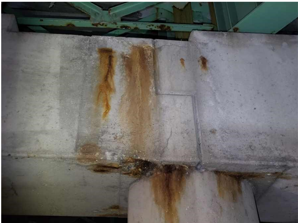
Photo 56: Pier cap, north face, above Column 3: spall and horizontal crack with efflorescence and rust staining.
