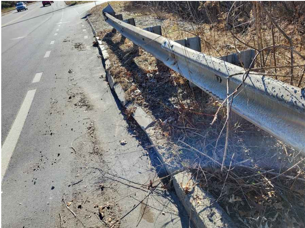
Photo 23: Southwest approach curb exhibits settlement and horizontal misalignment, up to 3" x 30' long. (Looking South).
