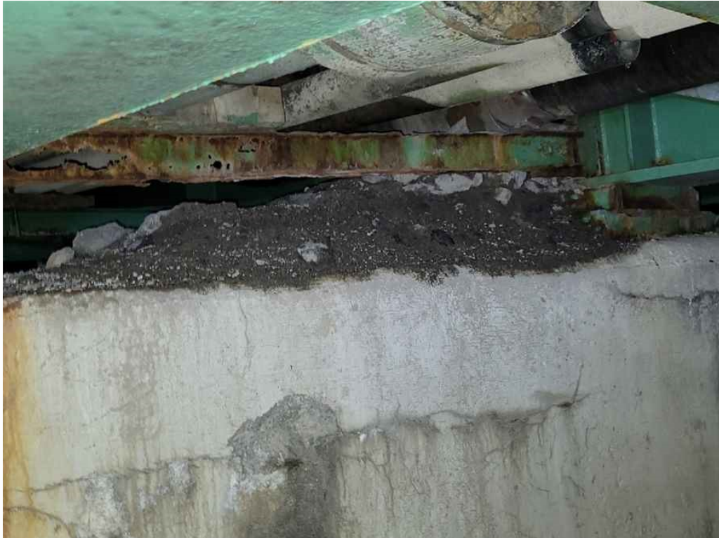
Photo 45: Bearings are partially covered by dirt and debris at the pier. (Bay 1, span 1 shown, looking North).
