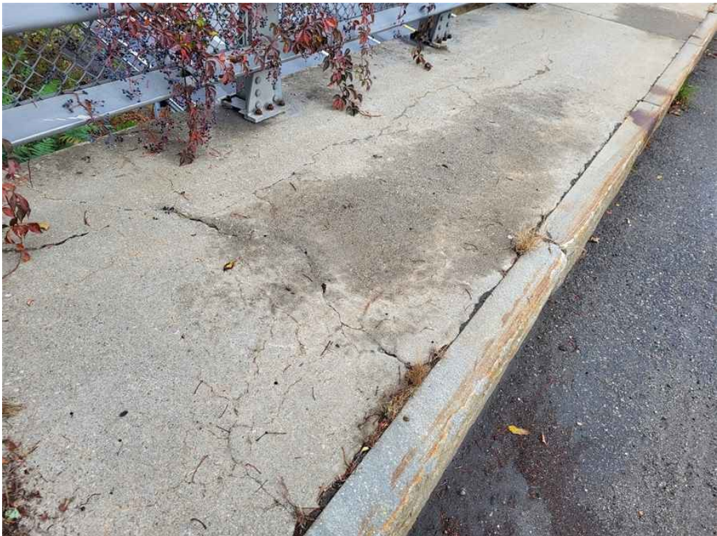
Photo 18: West Sidewalk: hairline transverse, longitudinal and map hairline cracking near the south end.
