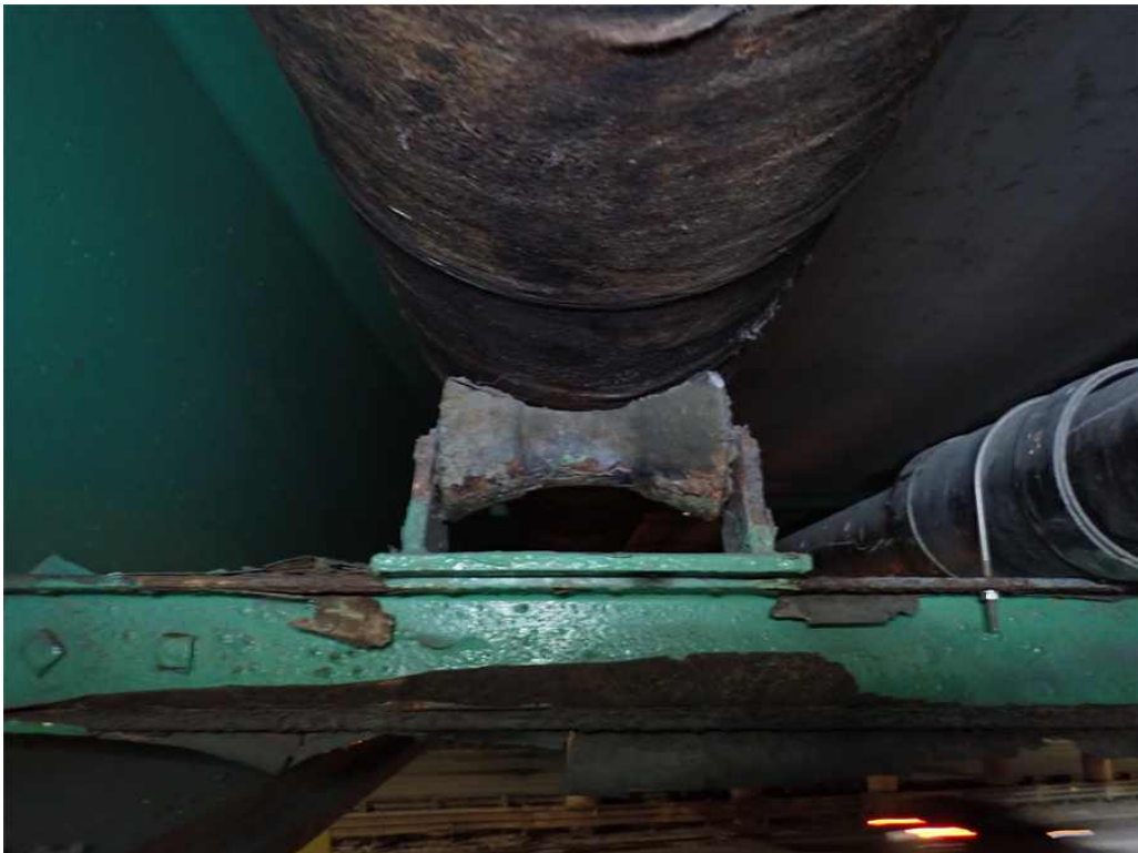
Photo 10: Typical area where the utility pipe is not seated properly in Bay 1 of Span 1.
