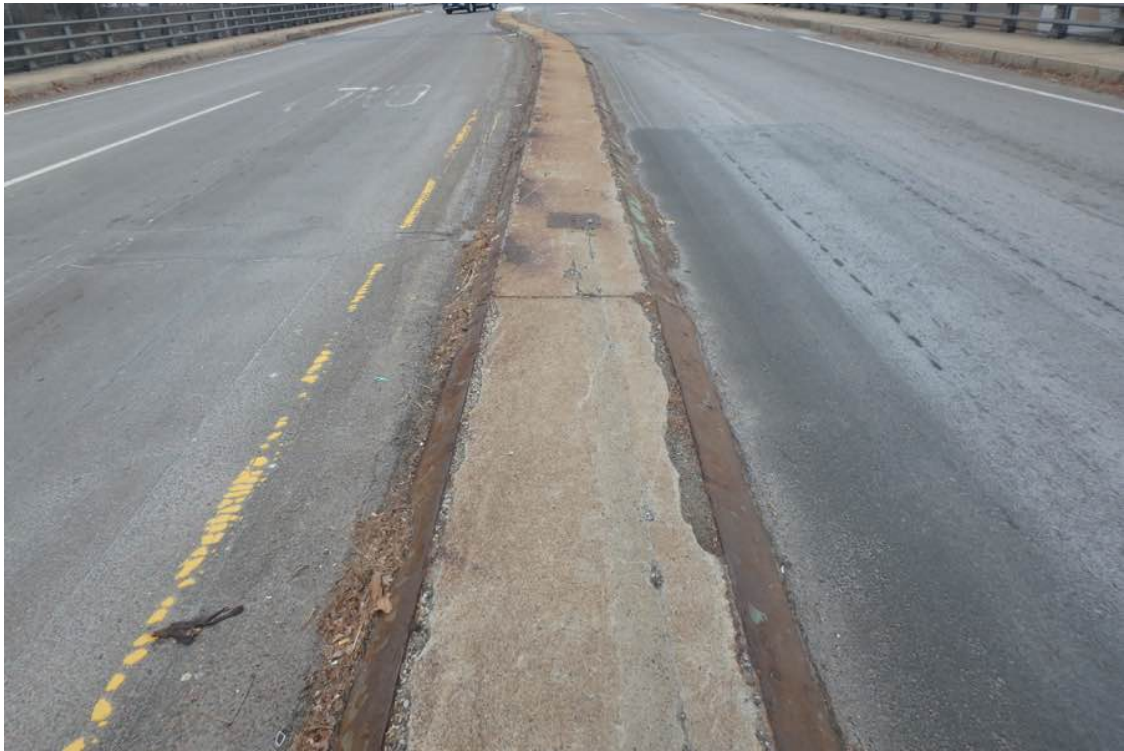
Photo 15: Typical spalling along both edges of the median; typical rust throughout the steel curbs.
