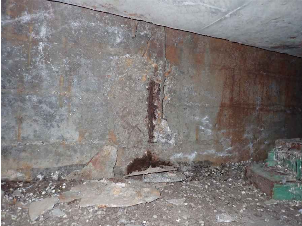
Photo 31: North Backwall behind in Bay 7 with spall and adjacent delamination.
