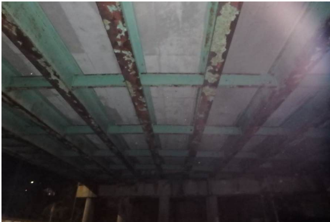
Photo 25: Typical rust and paint failure throughout all beams.
