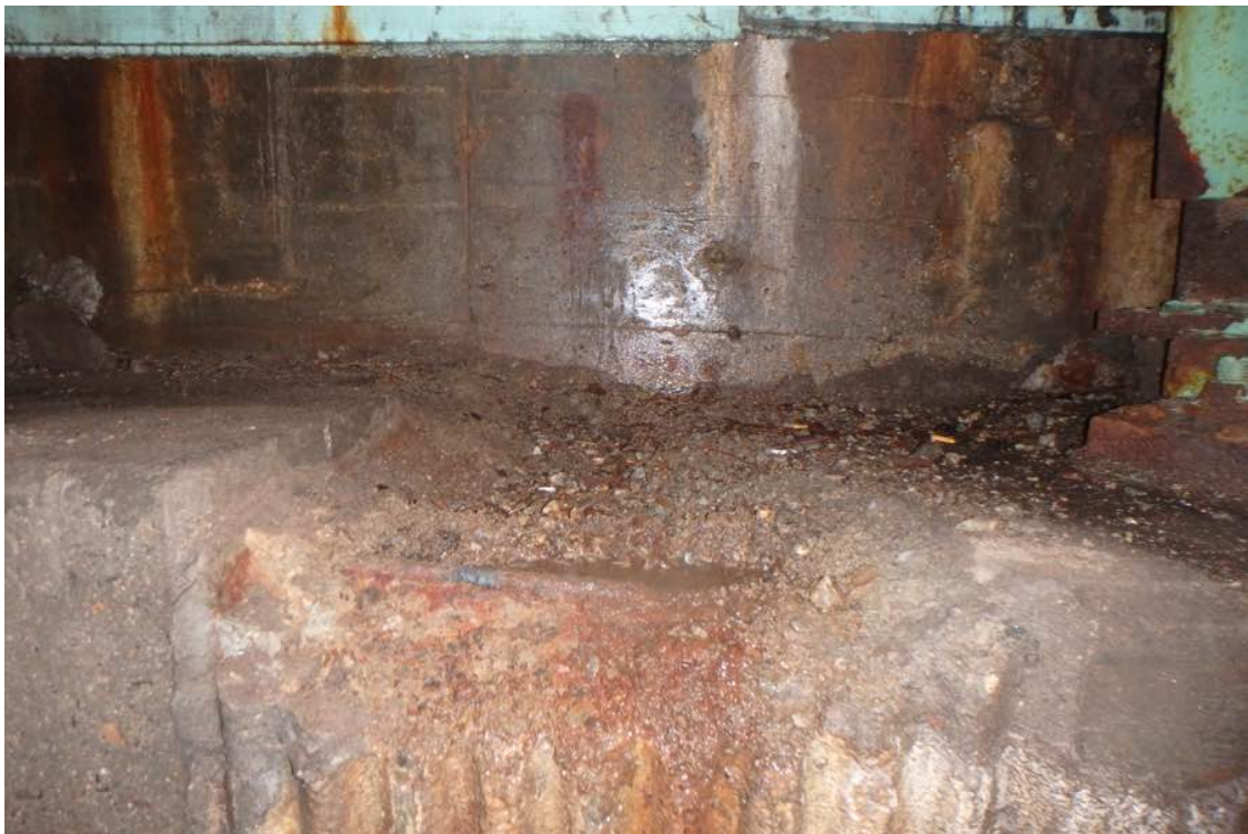
Photo 36: North breastwall, Bay 5 spalling.
