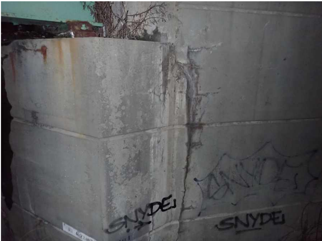
Photo 36: Northeast wingwall with vertical crack.
