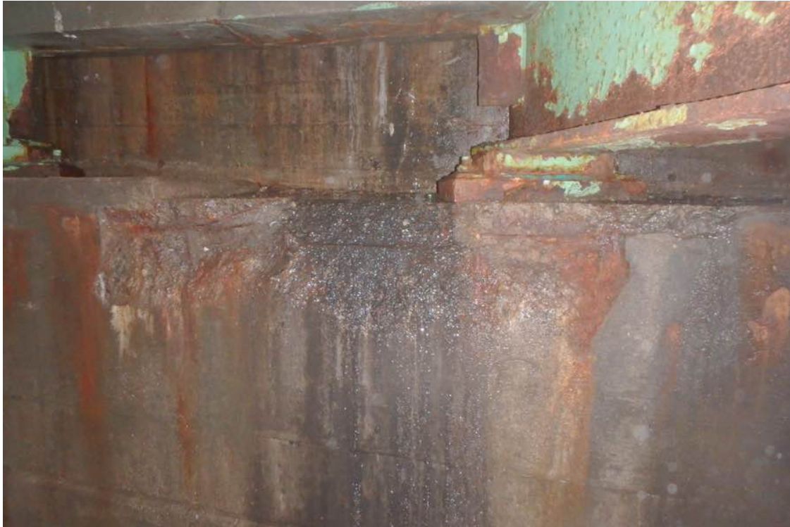
Photo 37: North breastwall, Bay 7 spalling.
