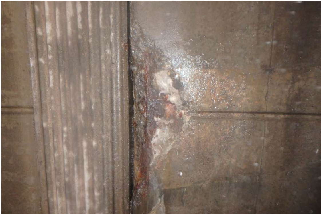
Photo 38: North breastwall, Bay 10 spalling.
