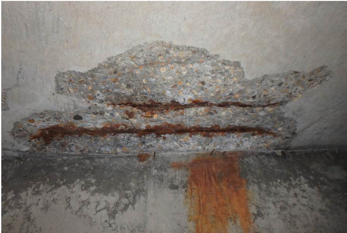
Photo 11: Span 2, Bay 8 spall over the pier.
