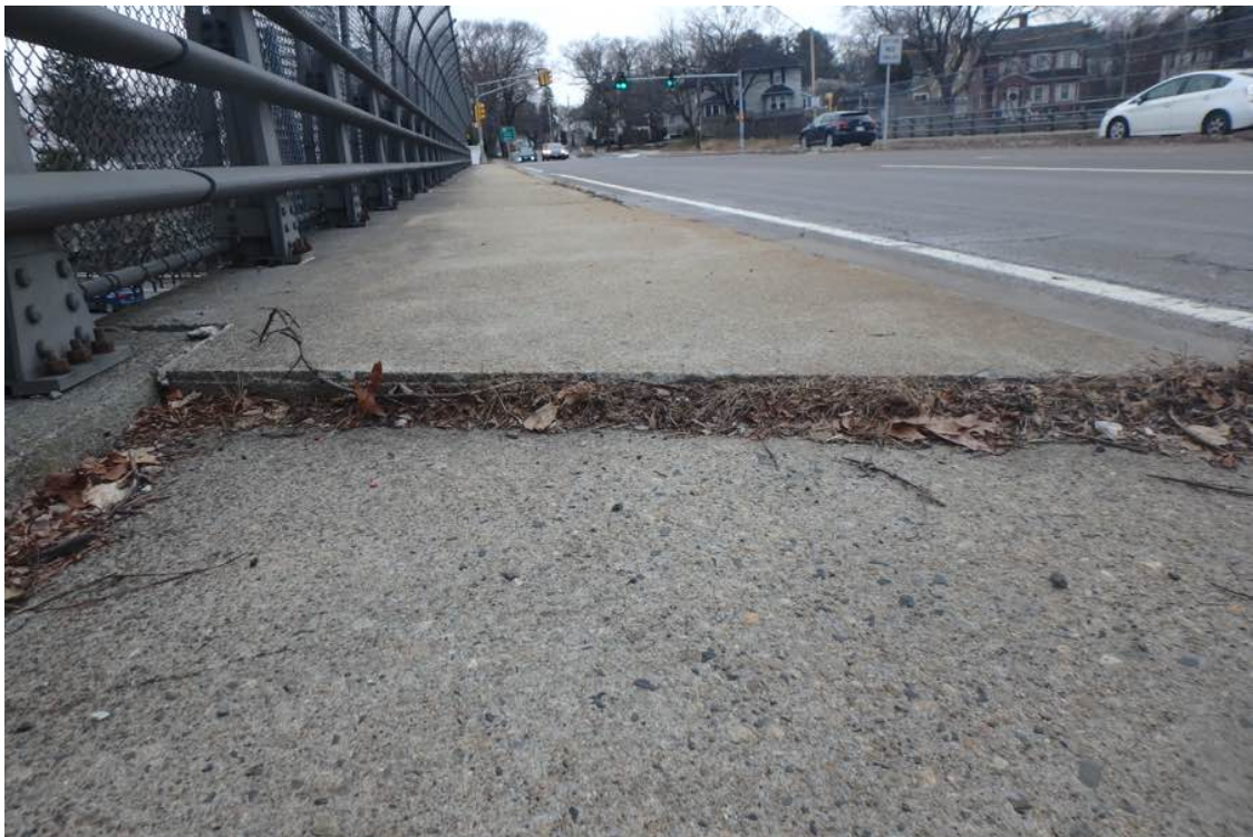
Photo 24: Southwest approach sidewalk settlement.
