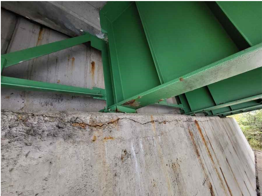
Photo 52: North breastwall: horizontal crack with minor rust staining under bays 3 - 5, up to 1/8" wide. (Looking East).
