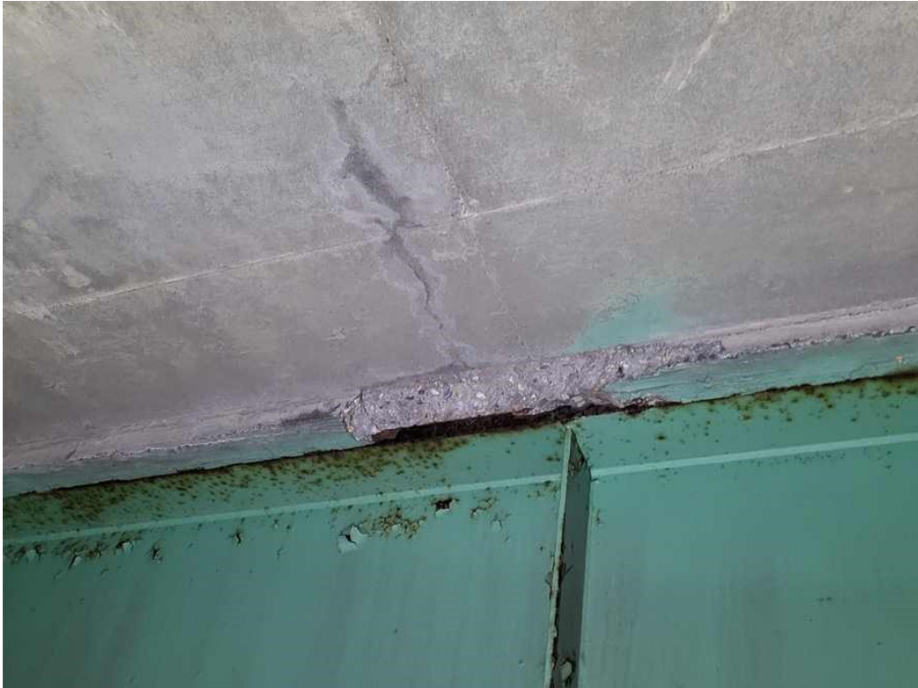
Photo 9: Deck, span 1, bay 5: between cross frames 3 and 4, 2' long x 1' wide x 2" deep haunch spall along Girder 6.
