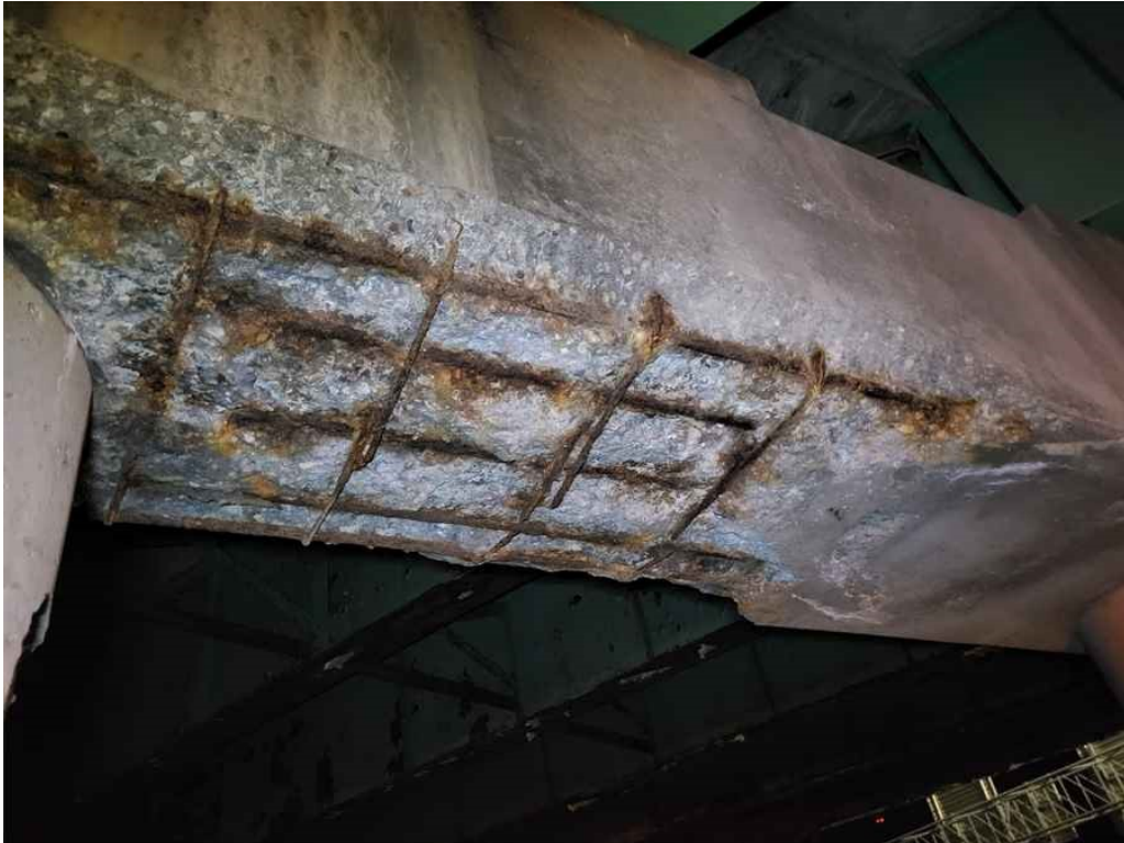
Photo 51: Pier cap, bottom Face, between Columns 1 & 2: sever spalling with exposed and broken rebar.
