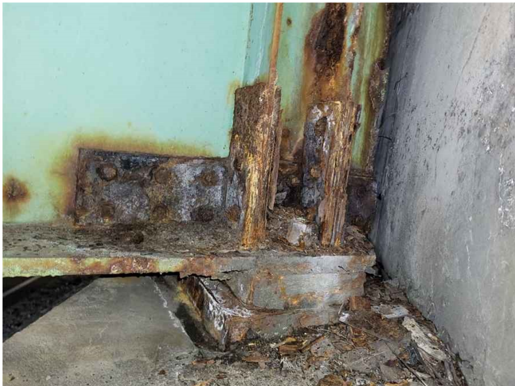
Photo 29: Girder 1: repair plates to the lower web and bearing stiffeners at the north abutment bearing with heavy rusting and minor steel delamination. Also note bearing rust. (East face shown).
