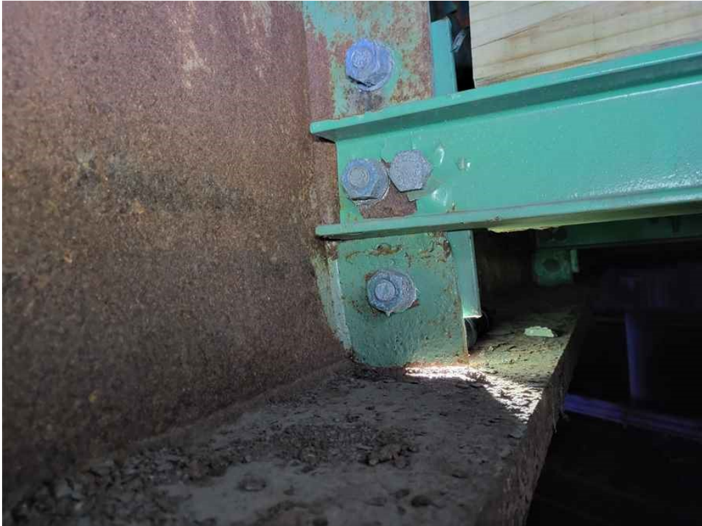
Photo 27: Girder 1, span 1: minor lateral misalignment of girder stiffeners and there is small gap between the stiffener bottom edge and the lower flange.
