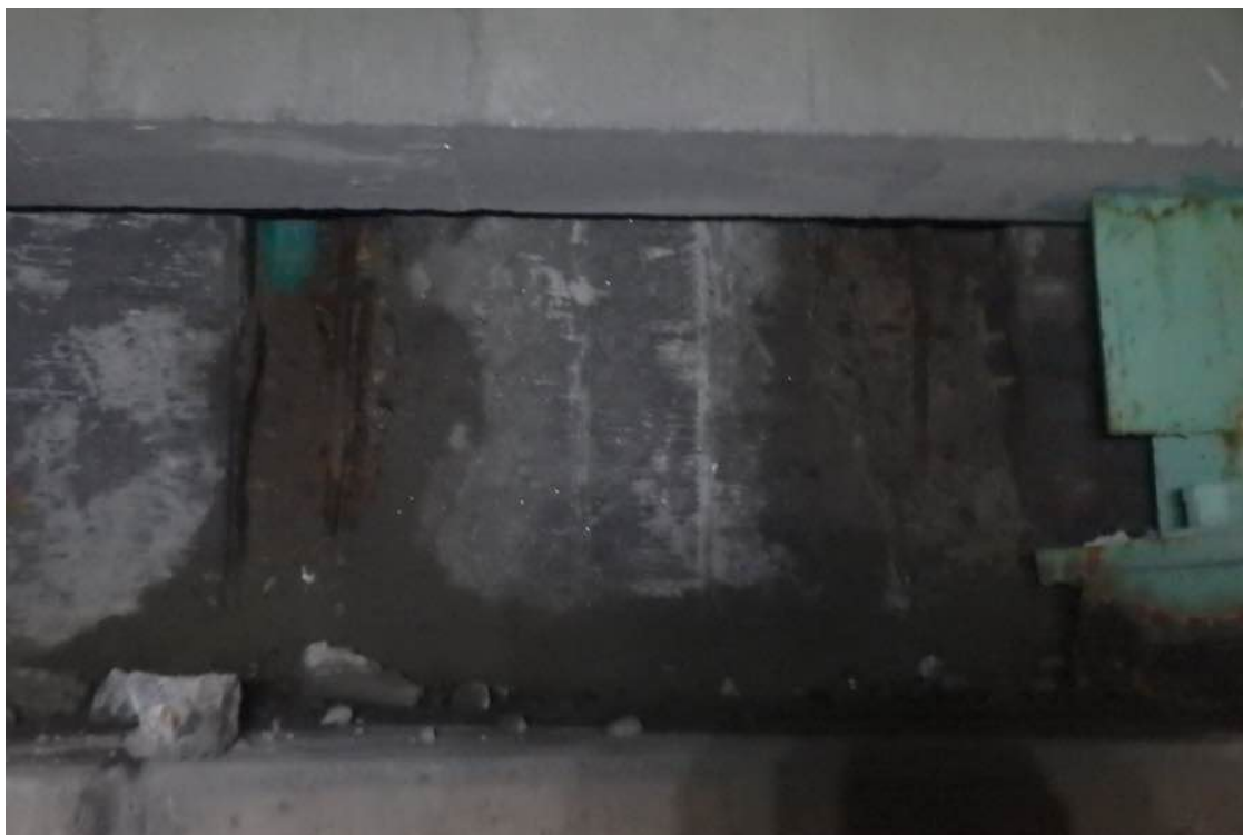
Photo 30: South backwall, full height spalling in Bay 2.
