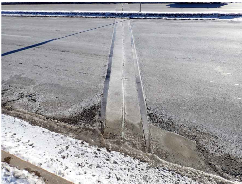
Photo 15: Pier joint in the southbound lanes.
