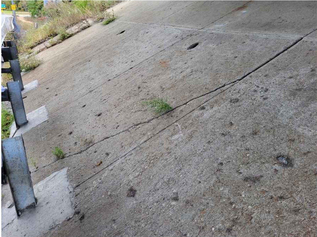
Photo 57: Slope paving at south abutment, under Bay 3: up to 1" wide diagonal crack at the bottom half.
