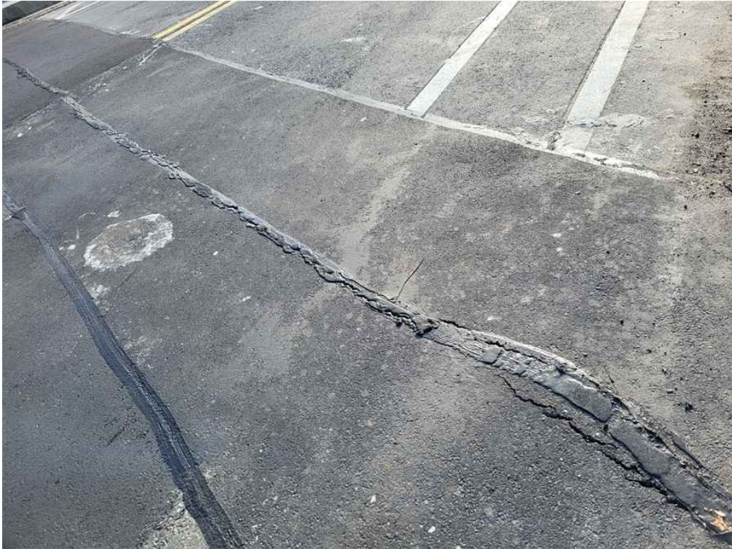
Photo 21: West end of south abutment deck joint exhibits up to 3' long x 1/4" transverse crack/separation.
