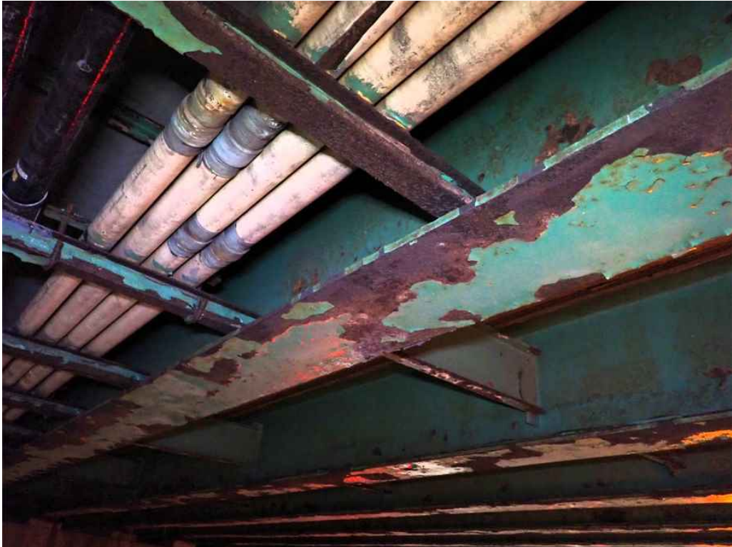
Photo 27: Typical paint peeling to the beams.
