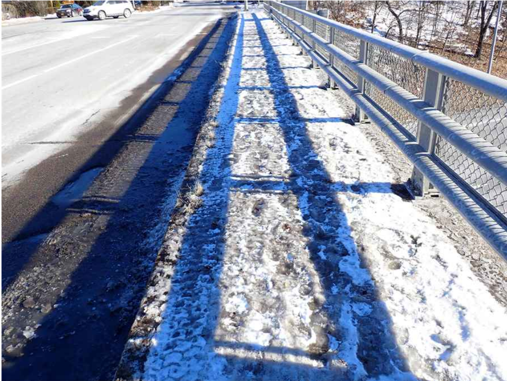
Photo 5: Both sidewalks are covered in snow and ice.
