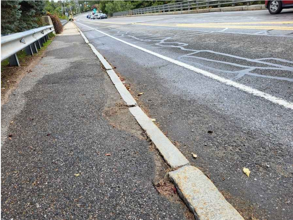
Photo 31: Southwest approach curb: vertical and horizontal misalignment, up to 3" and several areas of settlement. (Looking North).
