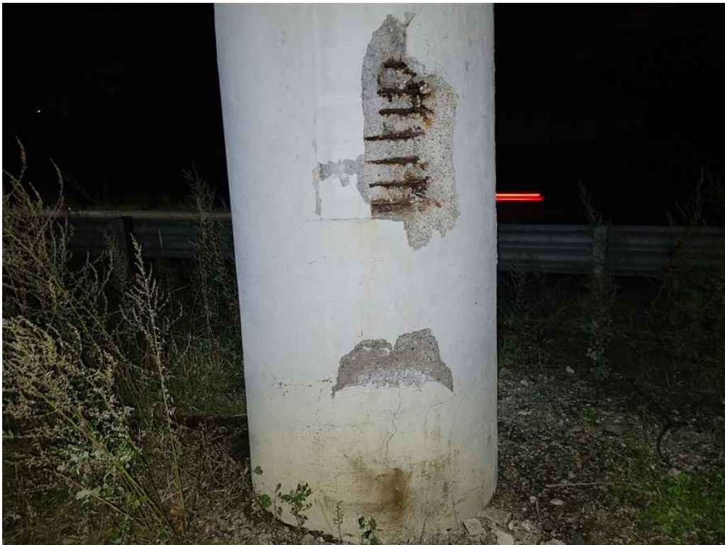
Photo 66: Column 1: several full height vertical hairline cracks, two spalls at the south face, up to 2' high x 1.5' wide x 3" deep with 7 exposed rebar.
