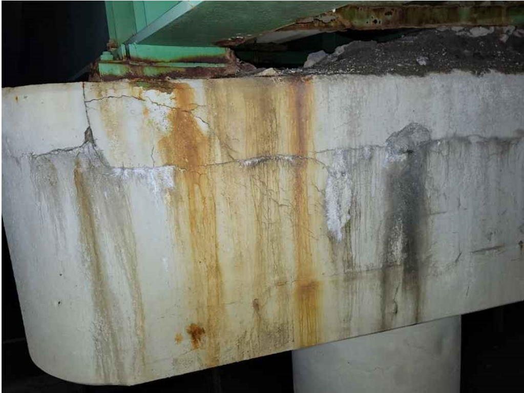
Photo 59: Pier, south face, bay 1, full bay length horizontal cracks, diagonal and vertical cracks under beam 1 with rust staining, up to 1/8" wide and up to 8" diameter x 1" deep spall.
