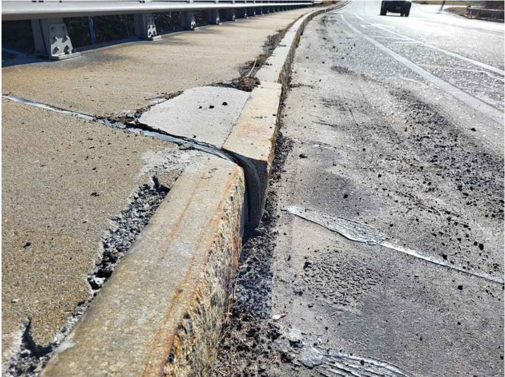
Photo 13: East granite curb at the pier deck joint is displaced and shifted 3" towards the roadway. Also, note the concrete repaired area at the sidewalk. (Looking South).
