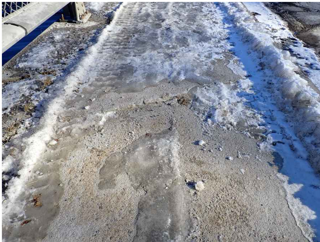
Photo 17: Southwest approach sidewalk settlement.
