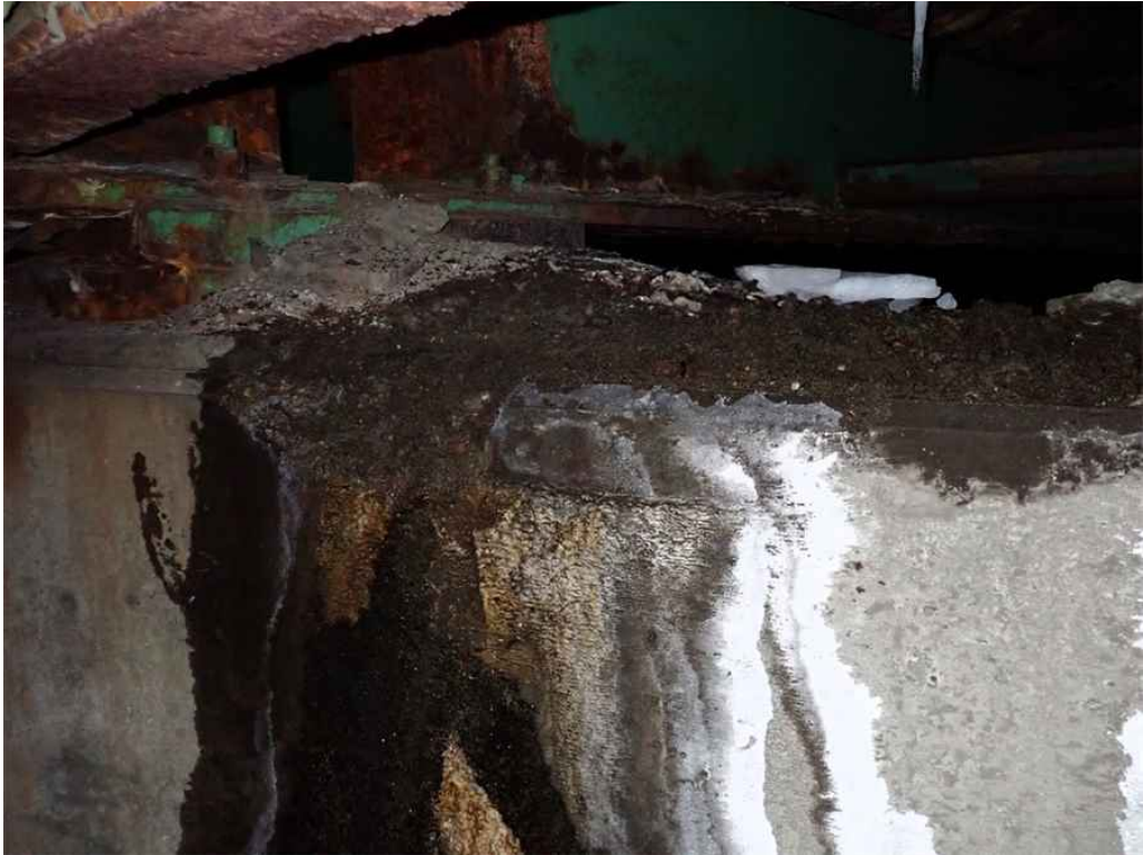
Photo 43: Pier cap, south face, below Bay 12 with spall along the top.
