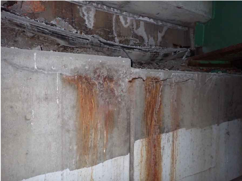
Photo 32: South breastwall with spall and exposed rebar along the top.
