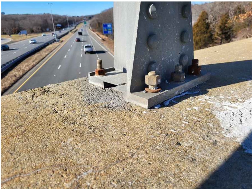
Photo 17: West safetywalk, Under-threaded bolt at post #10 from the pier in span 1.
