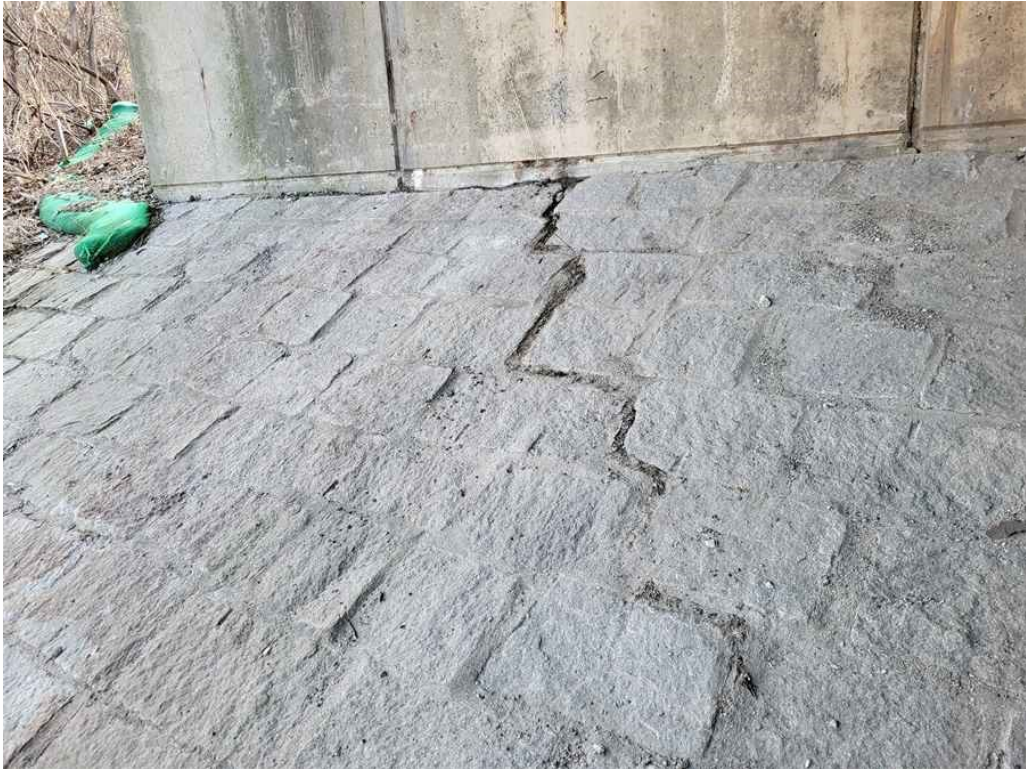
Photo 47: South stone slope protection: longitudinal crack through the pointing.
