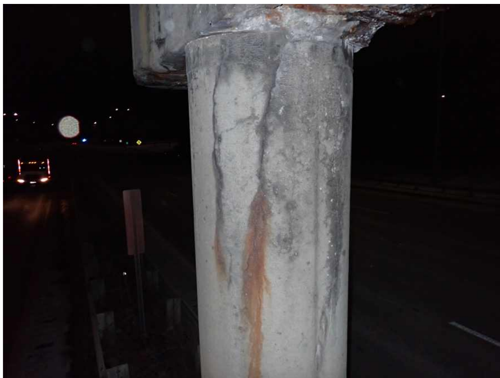
Photo 47: Top west face of Column 6 with delamination and vertical cracking.
