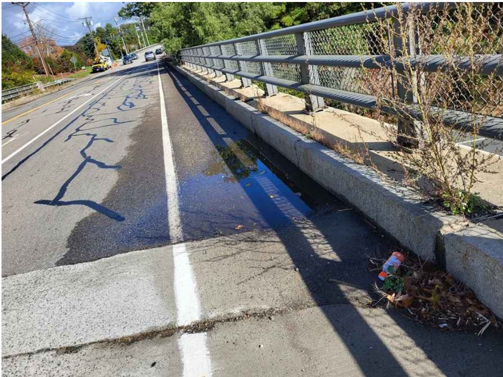
Photo 4: Wearing surface, span 1: area of ponding and standing water over the pier. (Looking North).
