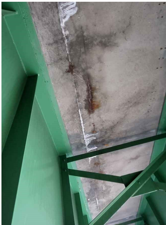
Photo 9: Deck, bay 4: full length delamination with moderate efflorescence, rust staining and dampness along the longitudinal construction joint.
