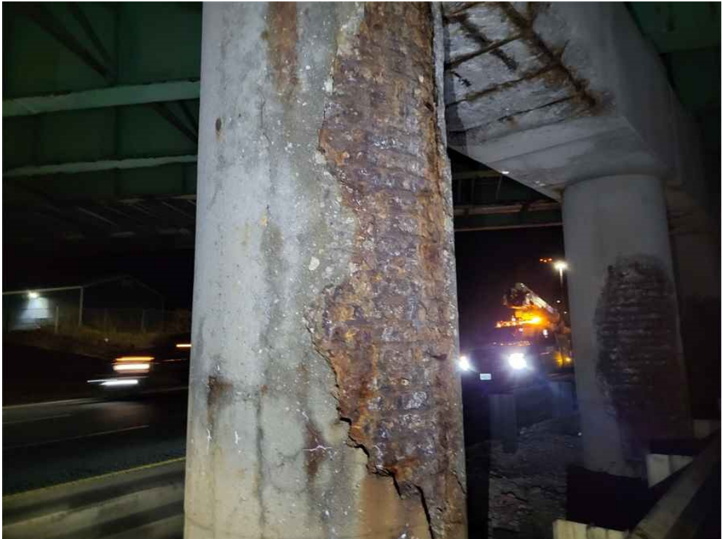
Photo 62: Column C4, south face: severe spalling throughout the south face, 8' high x 4' wide x 4" deep, with exposed rebar.
