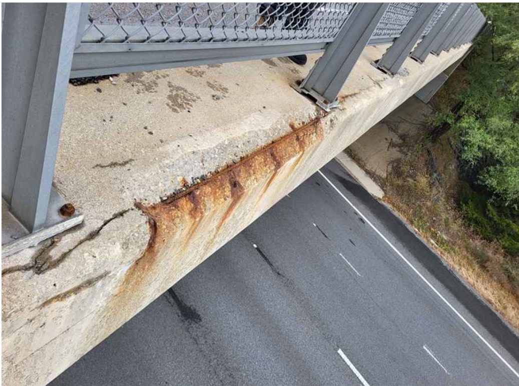
Photo 21: East safety walk: over the pier spall, 5' long x 5" high x 4" deep with exposed and rusted rebar along the outside edge.
