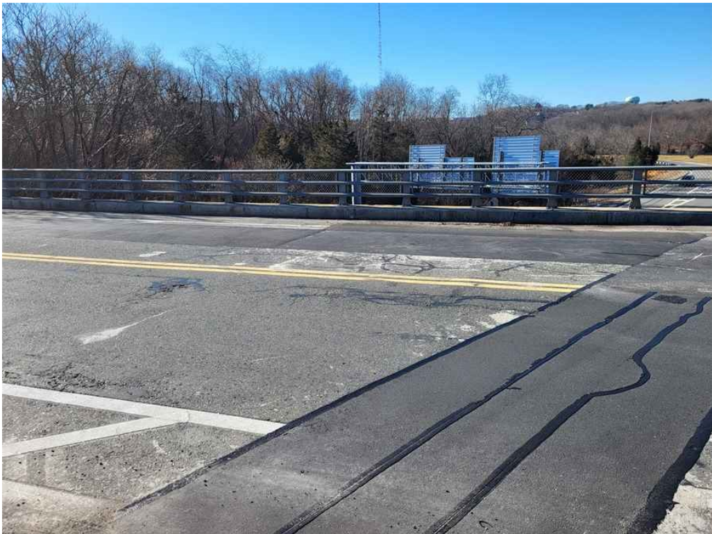
Photo 2: Wearing surface: full depth deck repair (20' long x 7' wide) in Span 2 of the southbound lane. (Looking West).
