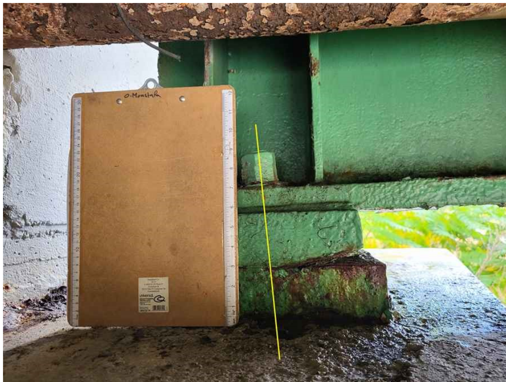
Photo 44: Bearing of beam 1, south abutment: east anchor is slightly bent towards the south.
