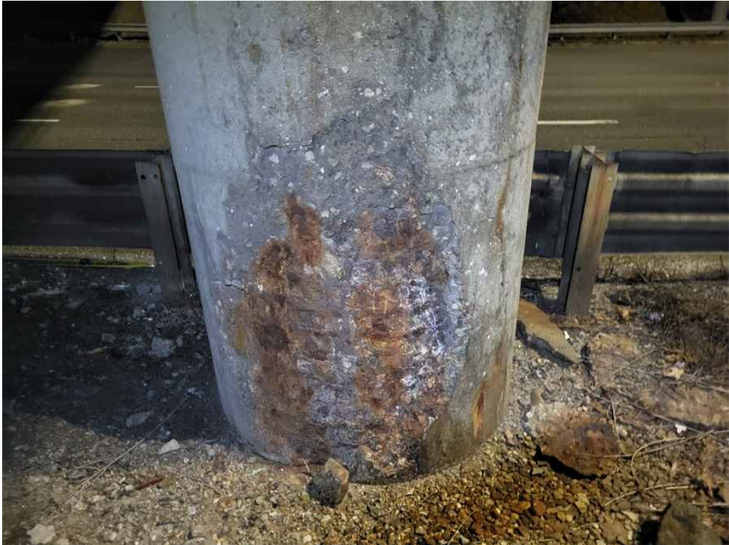
Photo 63: Column C4, north face: spall at the bottom, 3' diameter x 4" deep, with exposed rebar.
