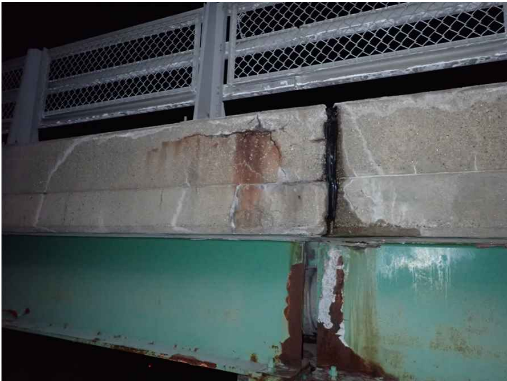
Photo 6: Delamination cracking to the outside face of the east sidewalk above the pier.
