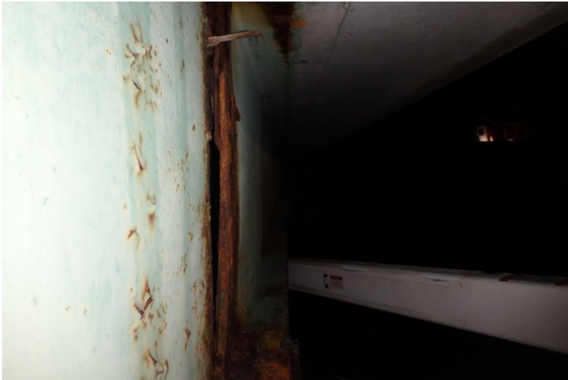
Photo 27: Span 2, Beam 211, deformation at the south end (Pier).
