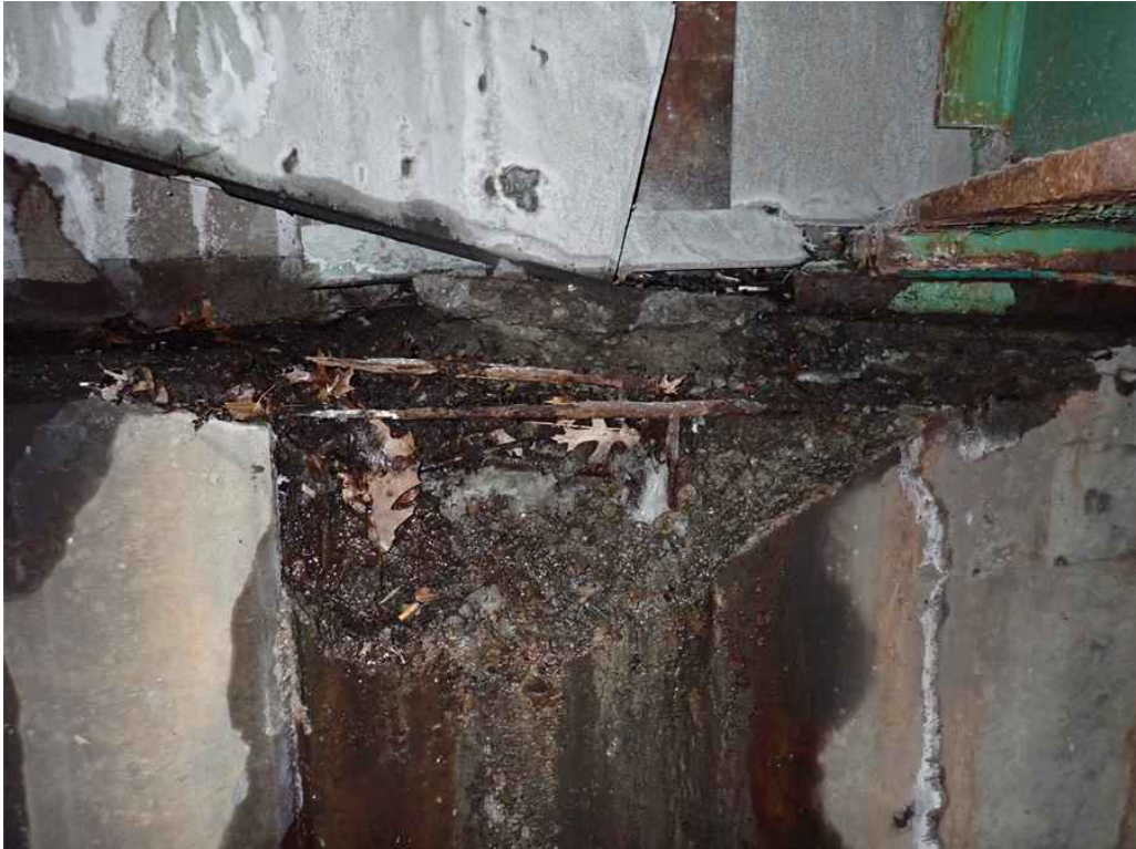
Photo 33: South Breastwall below Bay 11 with spall and exposed rusted rebar.
