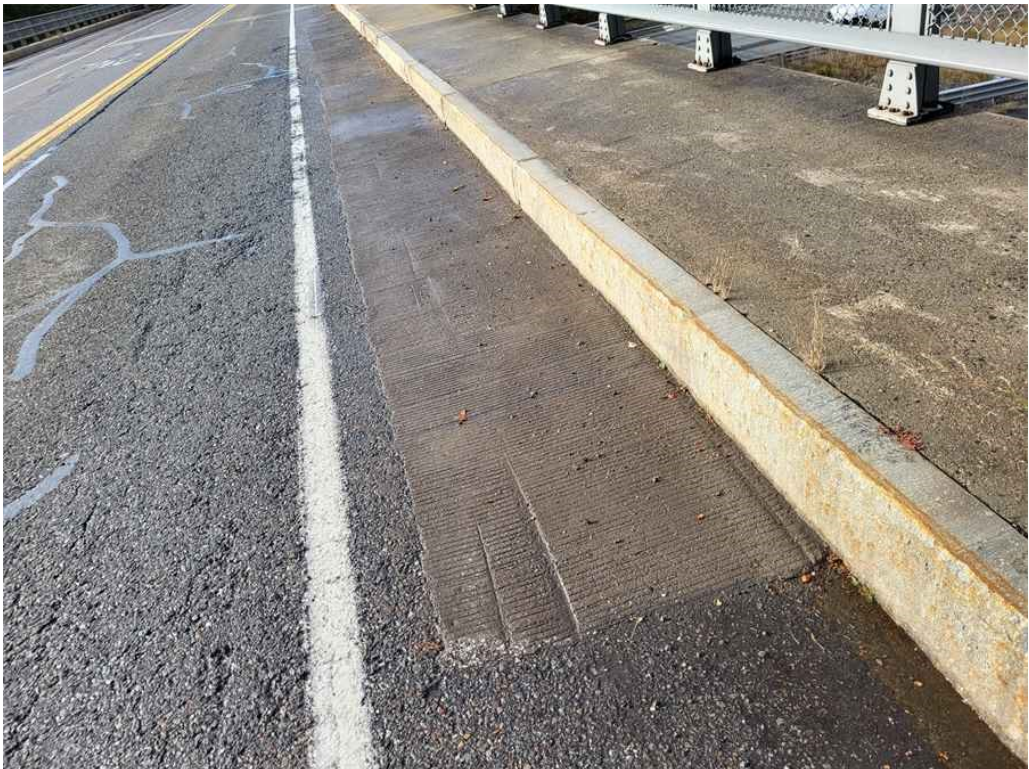
Photo 2: Wearing surface, Span 2, repair along the west curb. (Looking South).
