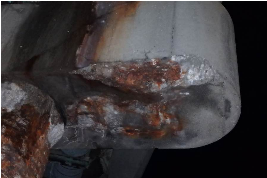
Photo 41: Pier cap, spall on the east nose.
