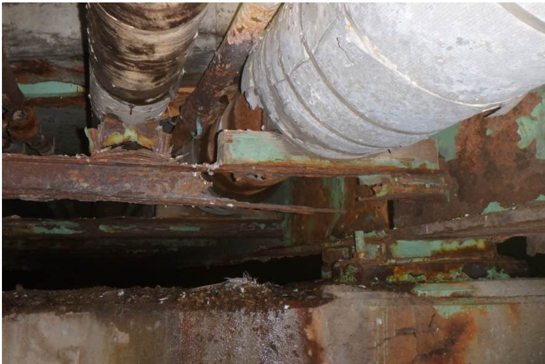
Photo 18: Bay 10 utility bracket at the pier joint with 100% section loss.
