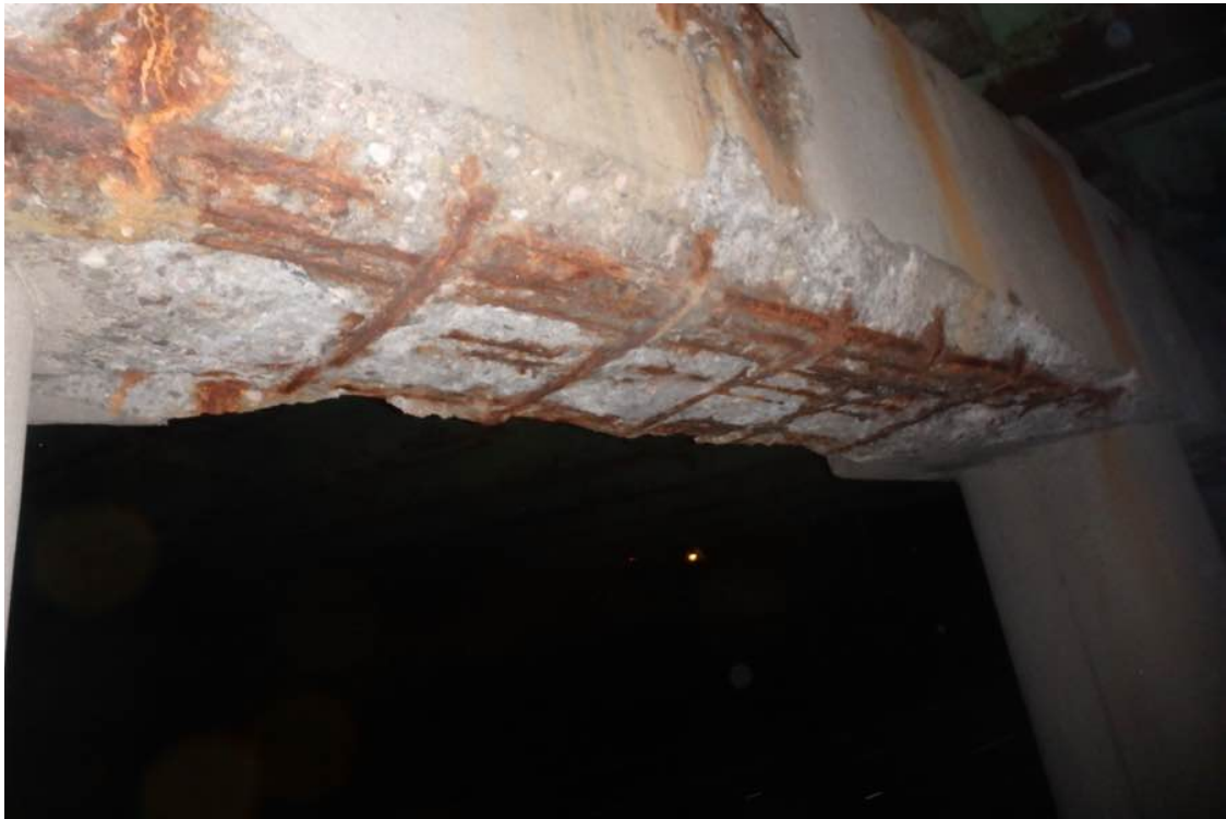
Photo 43: Pier cap, spall between Columns 2 & 3.
