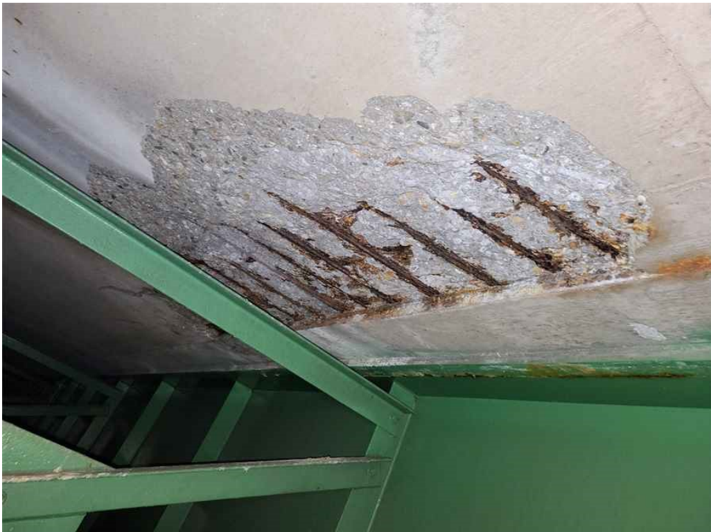
Photo 14: Deck, span 2 Bay 4, above the shielding: area of spalling, up to 32" wide x 7' long x 3" deep with 16 exposed/rusted rebar and adjacent hollow area, 3' long x 2.5' wide.
