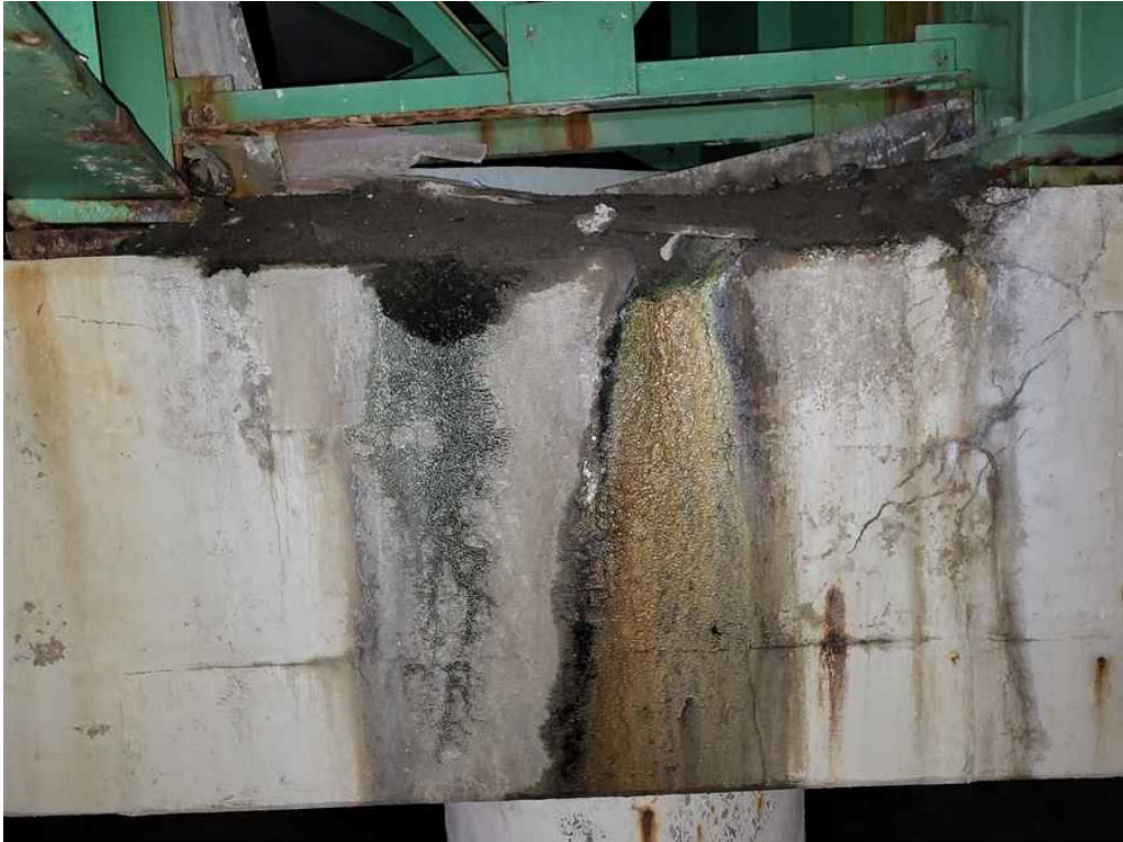
Photo 63: Pier cap, north face, bay 6, active leakage, moderate rust, efflorescence and a 9" wide x 4" high x 5" deep spall at the top. Also note the debris at the top of the pier cap.
