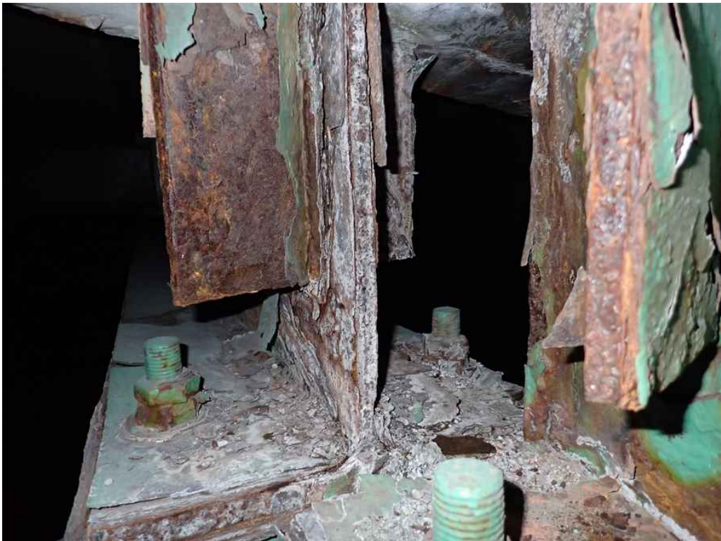
Photo 22: Beam 206 at the pier with rusting, section loss and slight bent to the bottom of the web.
