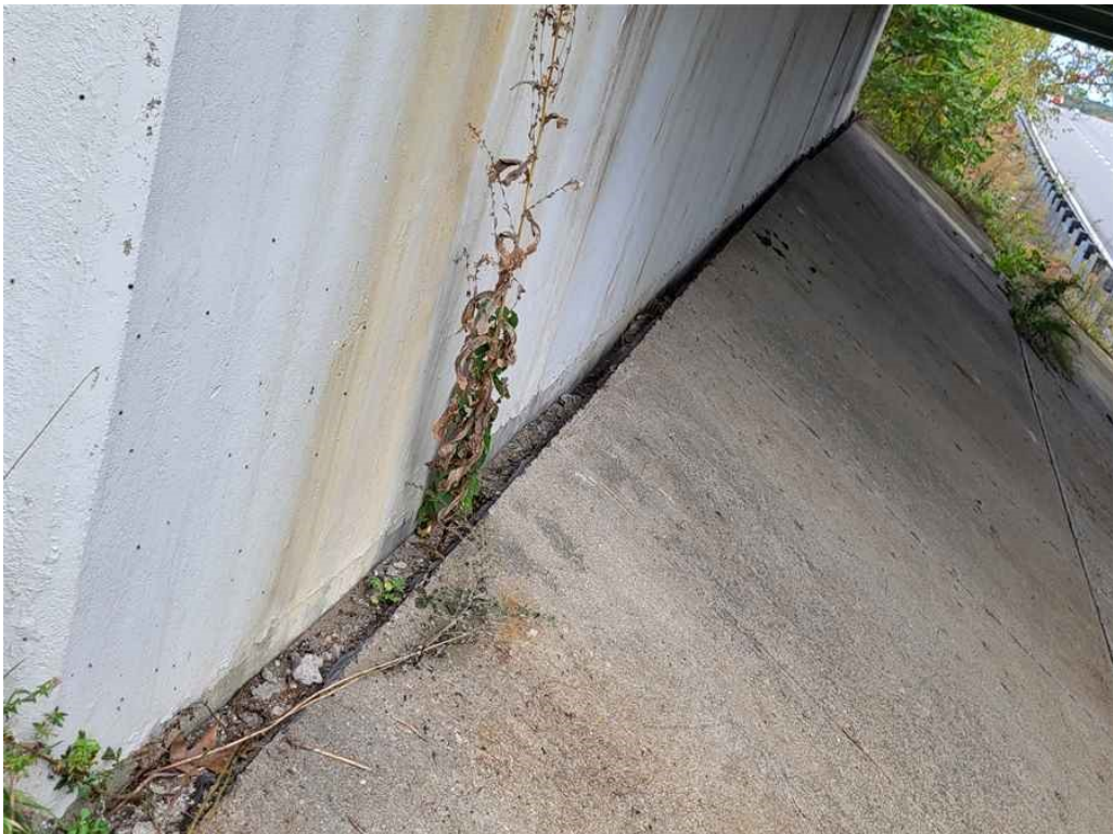
Photo 56: Slope paving at south abutment: 3" to 4" wide gap at the top of the slope pavement.
