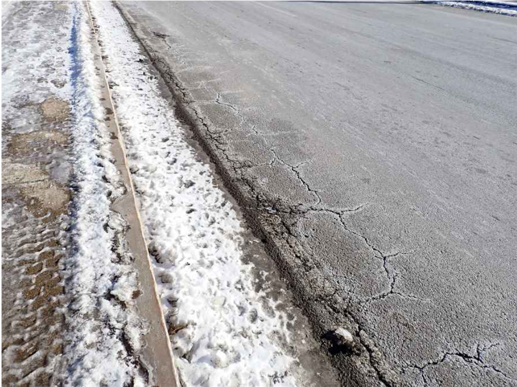
Photo 1: Wearing surface with map cracking along the west curb.
