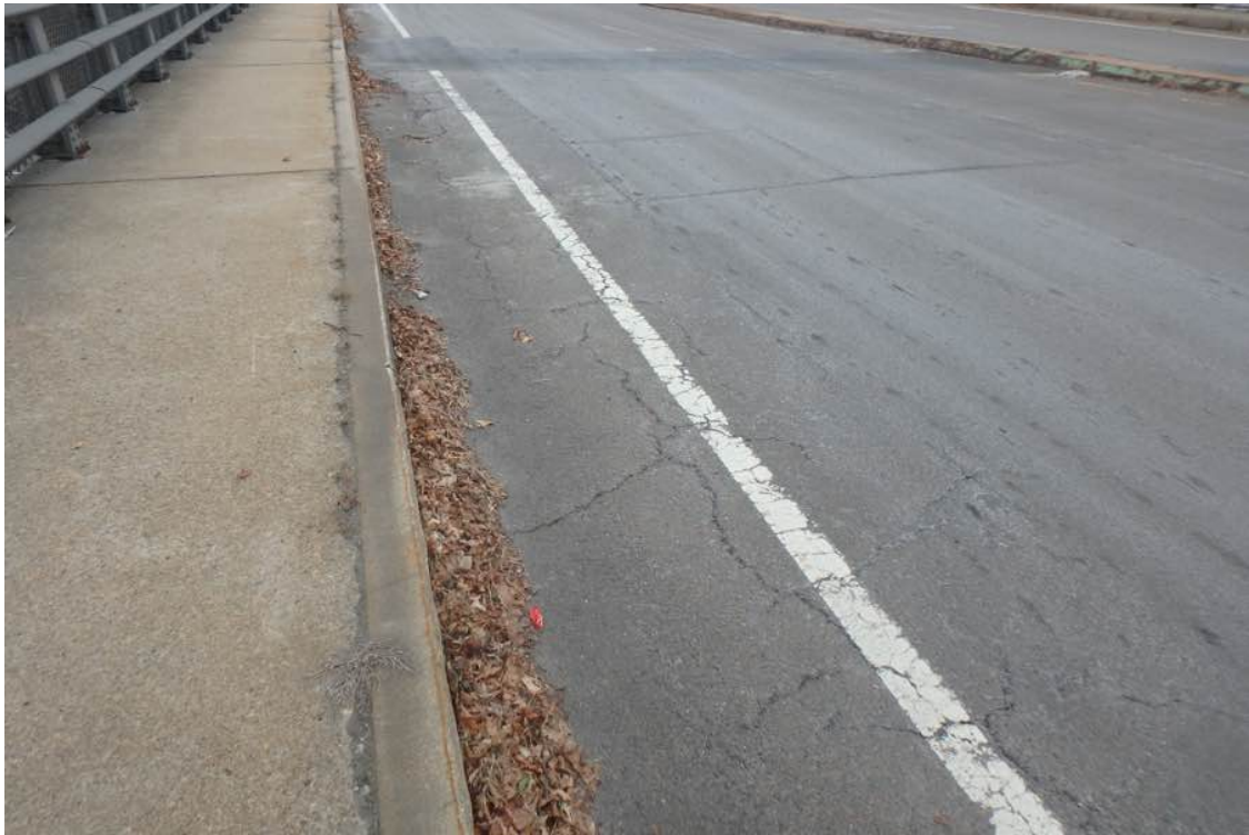
Photo 1: Wearing surface, typical cracking along the fog line in both spans.
