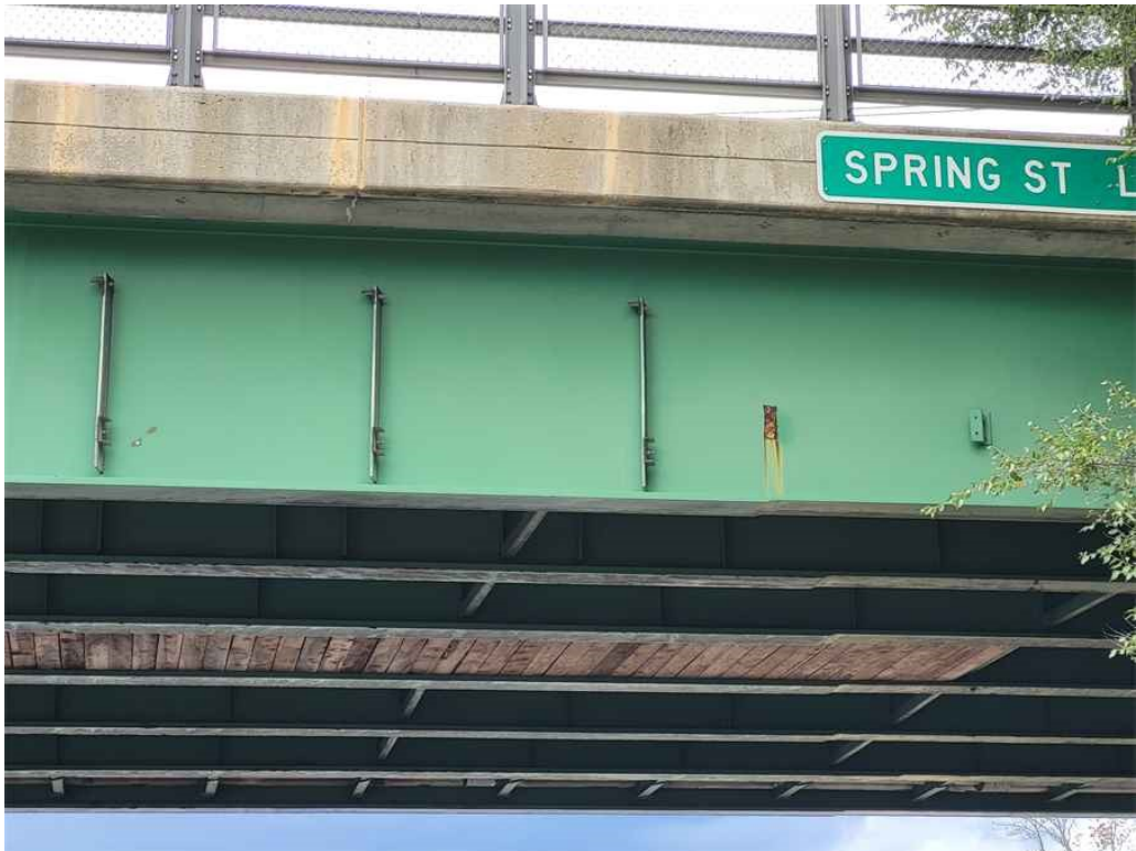
Photo 40: Span 2, beam 14, east face has abandoned brackets.
