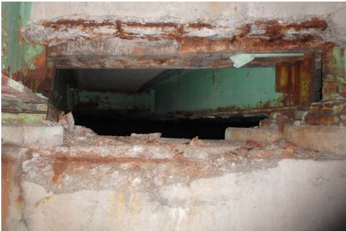
Photo 48: Pier cap, spall between Beams 208 & 209.
