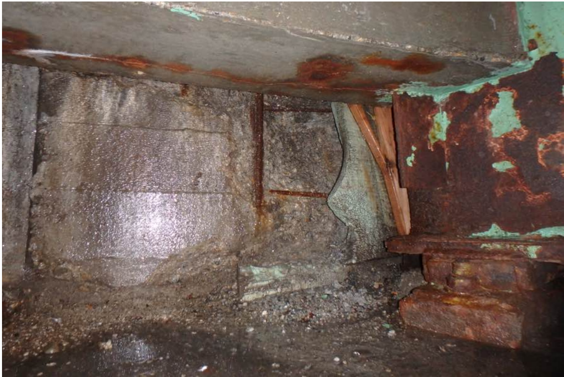
Photo 31: North backwall, Bay 9, spalling behind Beam 210.
