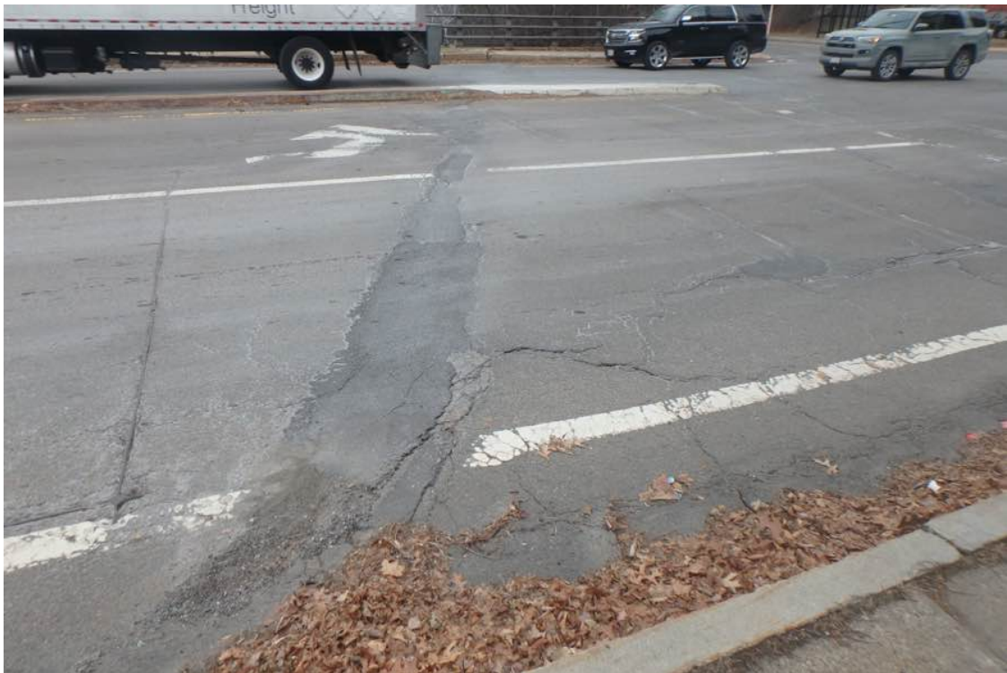
Photo 2: Southbound roadway, deterioration along the south deck end.
