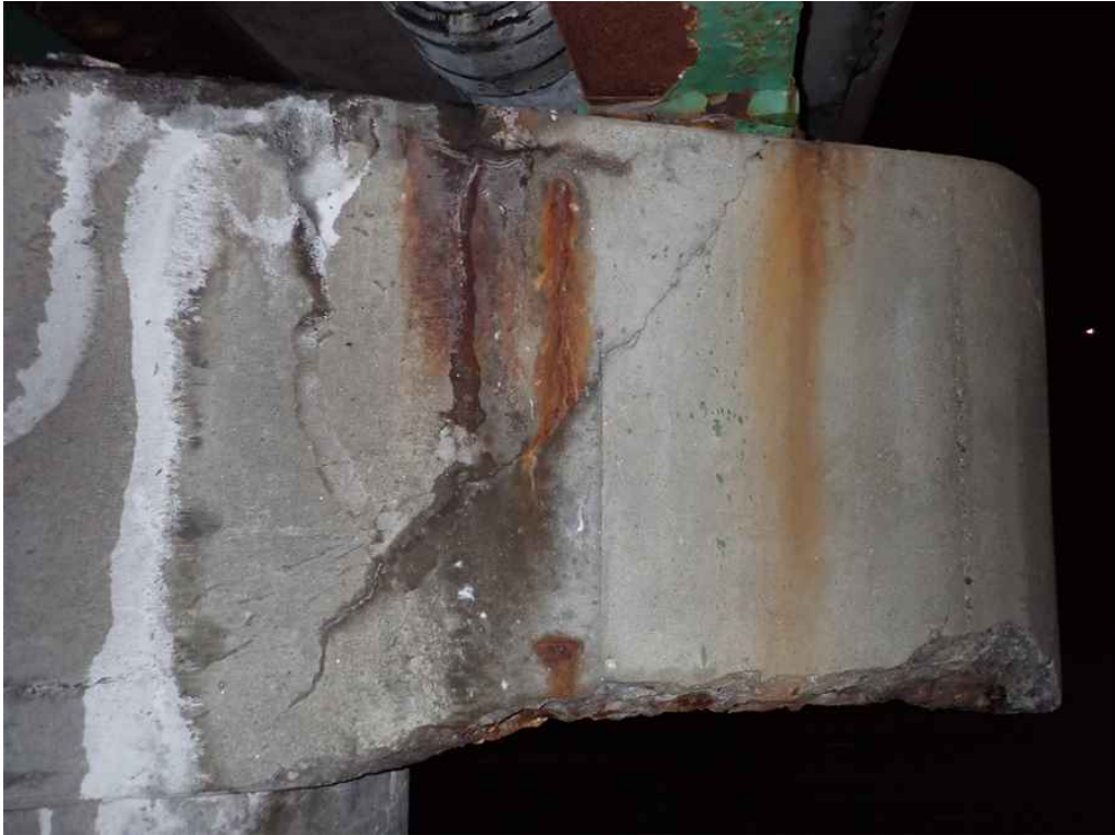
Photo 45: Pier cap, south face, east end with diagonal crack.
