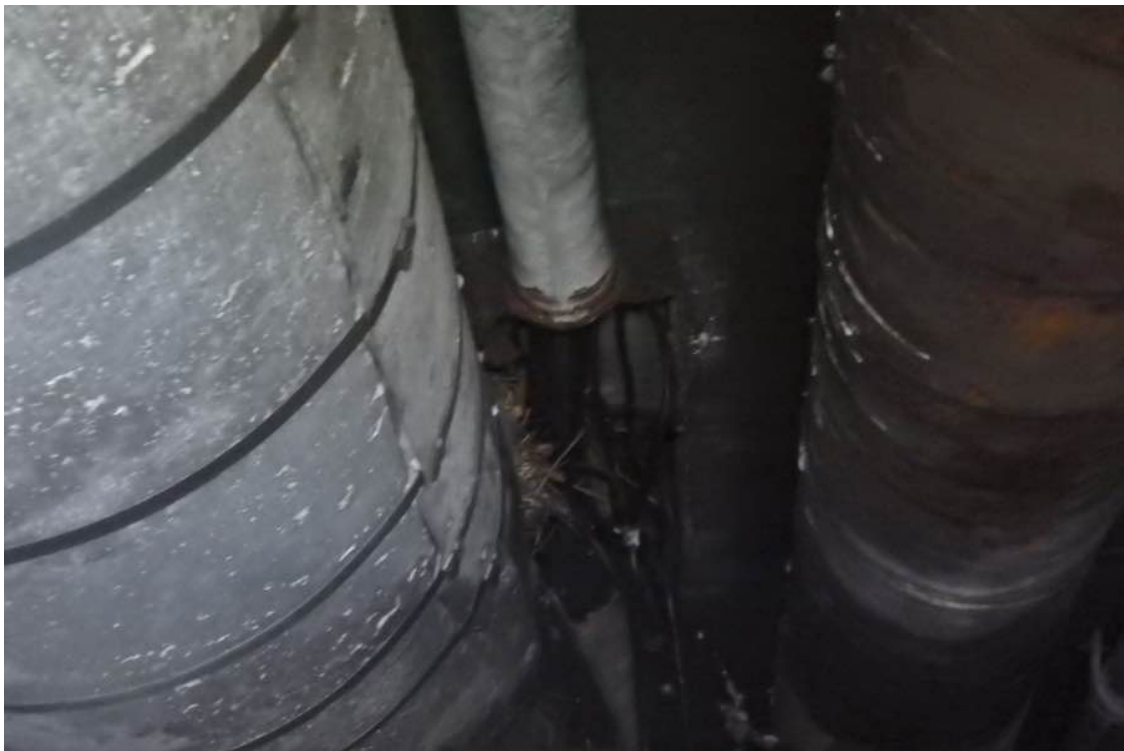
Photo 22: Span 2, Bay 10 utility hand-box rusted through with exposed wires.
