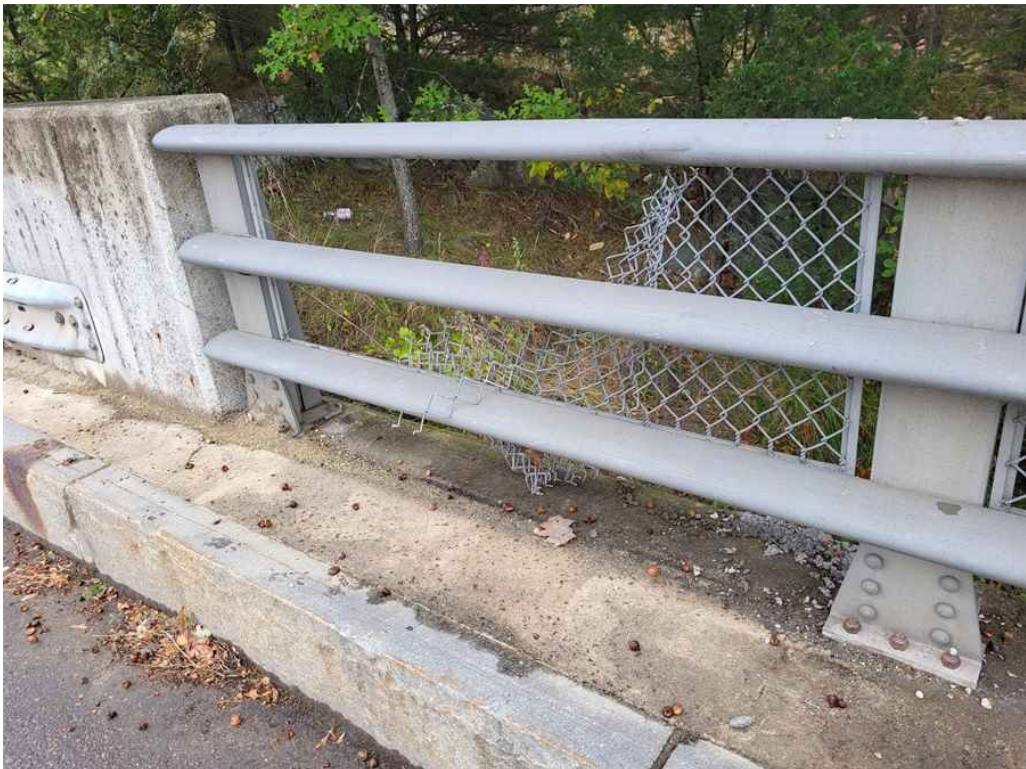
Photo 24: The metal fencing is detached at the first panel from the north in the east railing.
