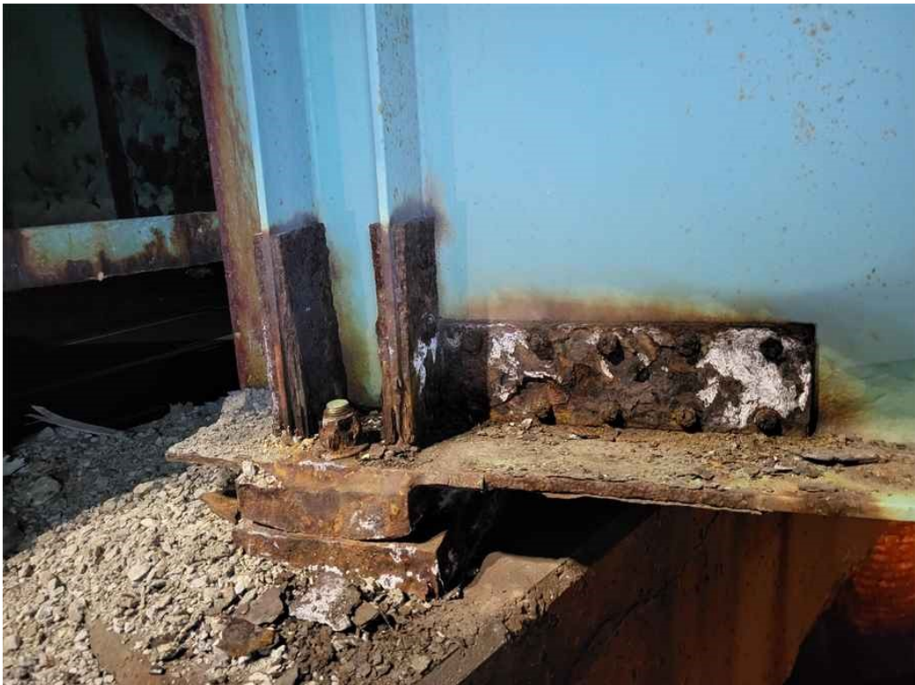
Photo 36: Girder 14, span 2 at the pier: repair plates on both sides of the lower web and bearing stiffeners that exhibit heavy rusting. Also note bearing rust. (East face shown).
