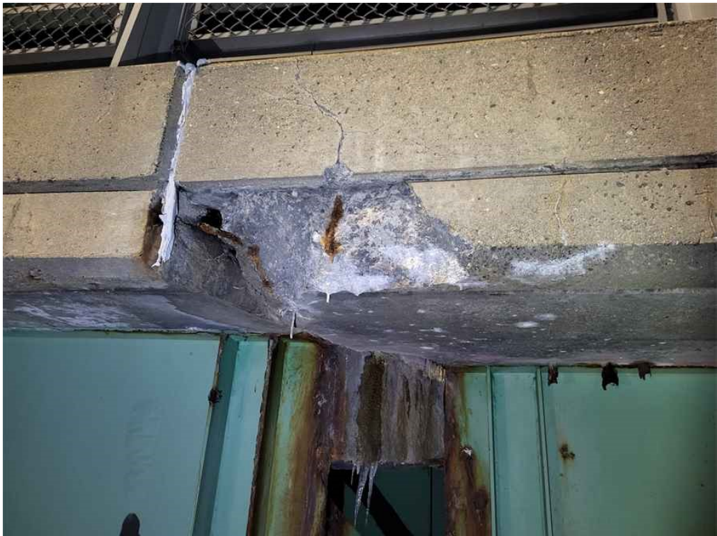
Photo 12: Deck, span 2, west overhang: 2' long x 8" high x up to 12" deep spall with exposed rebar at the pier.
