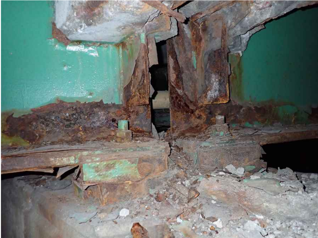
Photo 21: Beams 102 and 202 at the pier, east face, with rusting and section loss.
