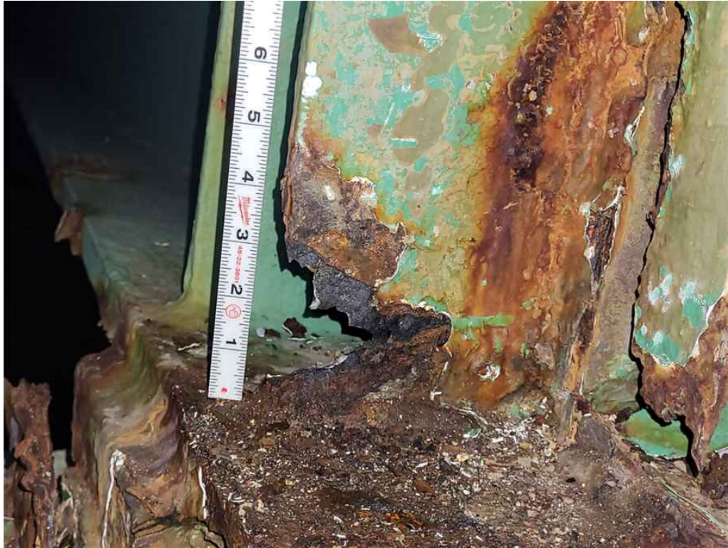
Photo 39: Beam 7, span 1: east stiffener at the very end has an area of 100% section loss, 3" wide x 2" high.
