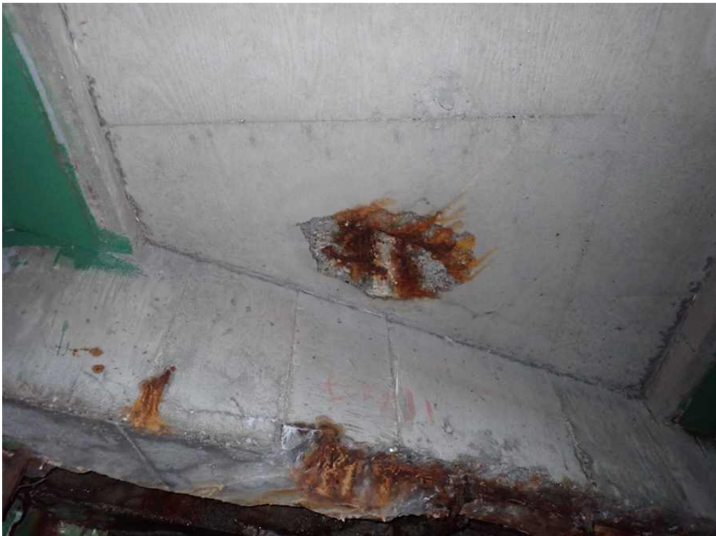
Photo 2: Spall to the deck at the north end of Bay 11 in Span 1.
