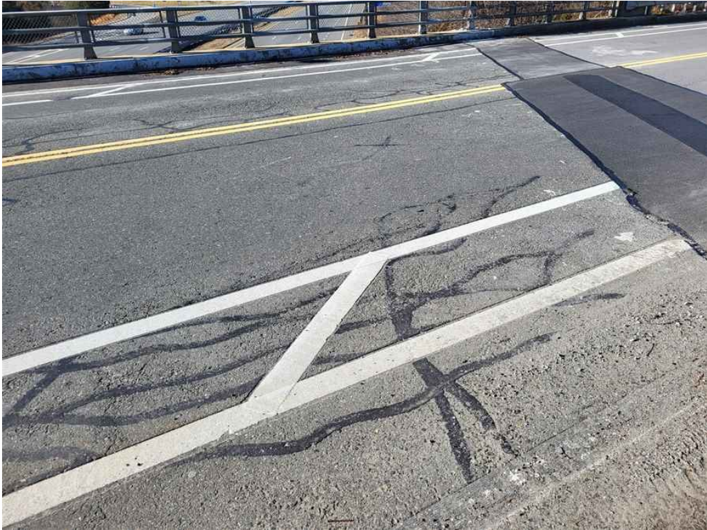
Photo 1: Wearing surface: random sealed cracks throughout. (Span 1, looking South).
