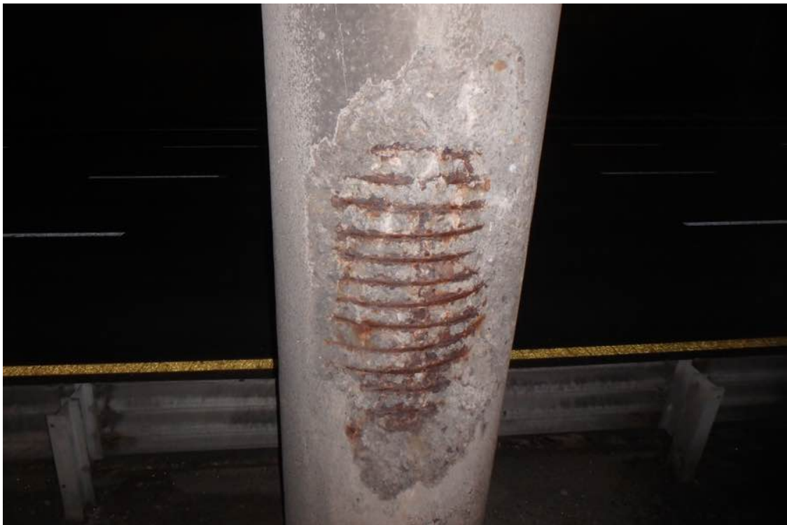
Photo 50: Column 2 spall on the north face.
