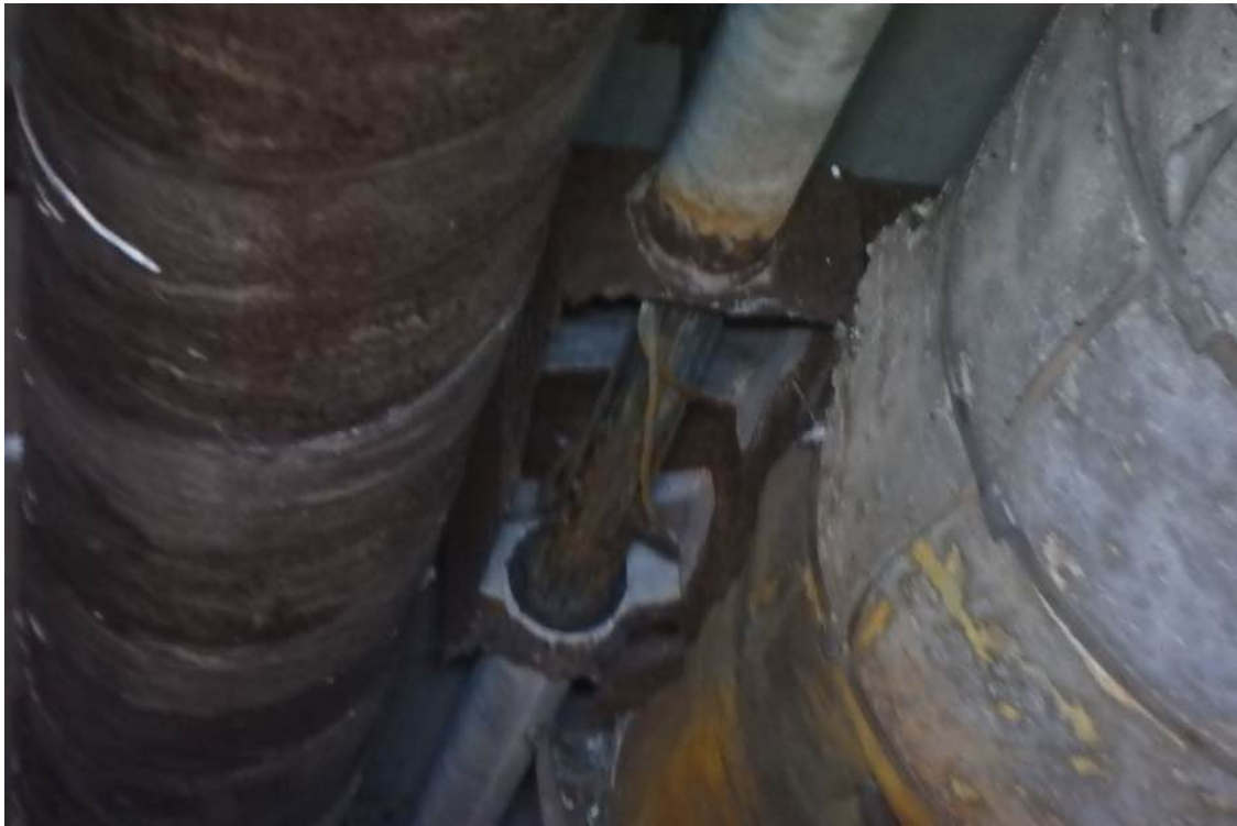
Photo 21: Span 1, Bay 10 utility hand-box rusted through with exposed wires.
