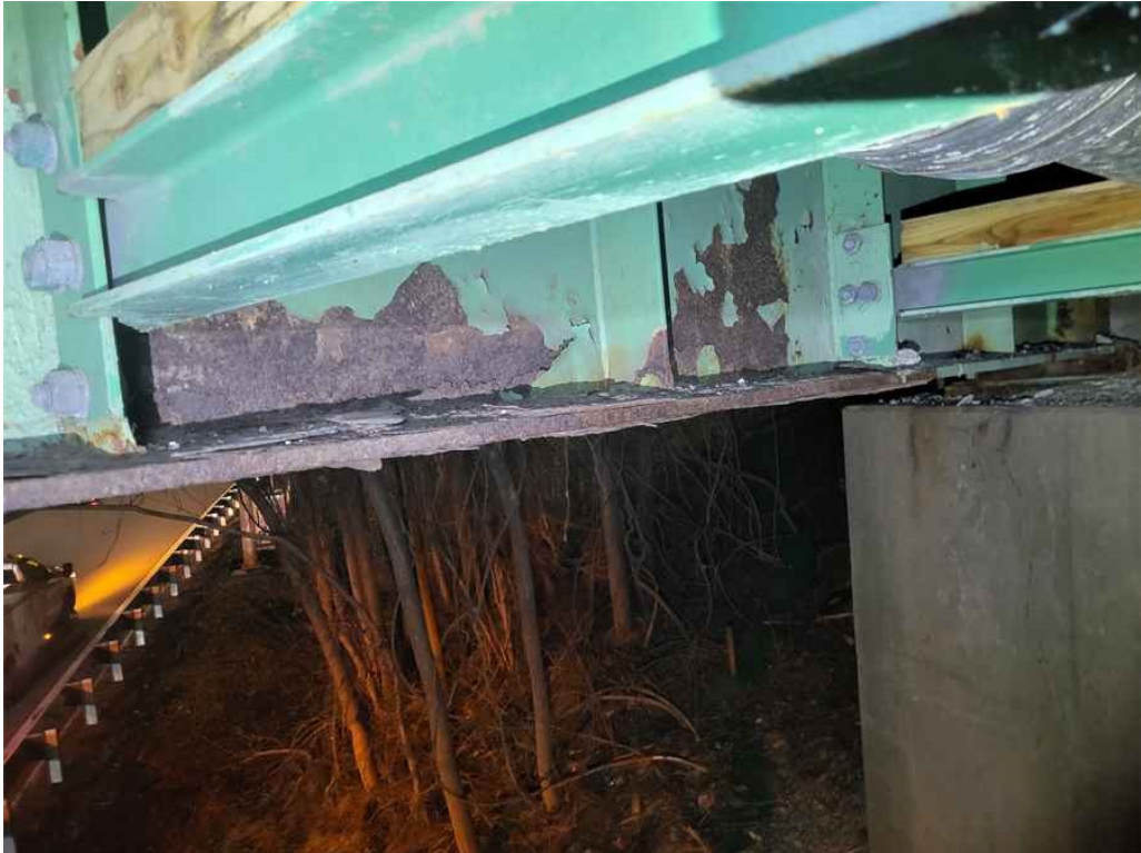
Photo 35: Girder 8, south end with minor section loss to the west face of the web. The west leg of the bottom flange exhibits heavy lamination with 3/16" section loss over a length of 7'.
