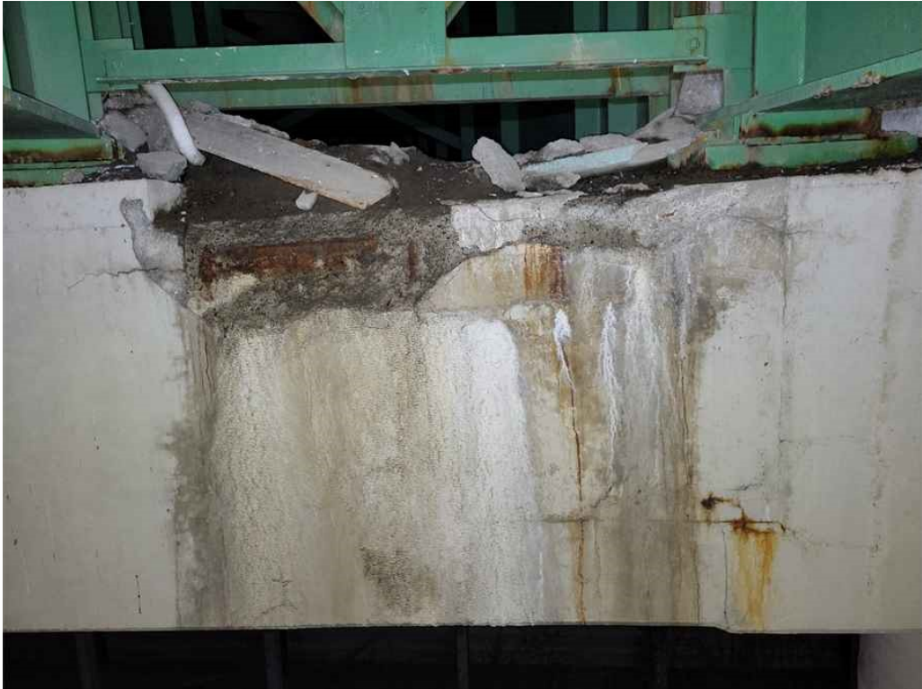
Photo 61: Pier cap, south face, bay 5, two spalls at the top, up to 3' wide x 1.5' high x 3" deep with exposed rebar and a 1/4" wide horizontal crack between the spalls.
