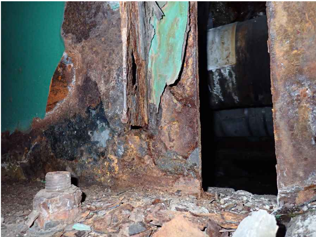
Photo 24: Beam 212 at the pier with rusting and section loss.
