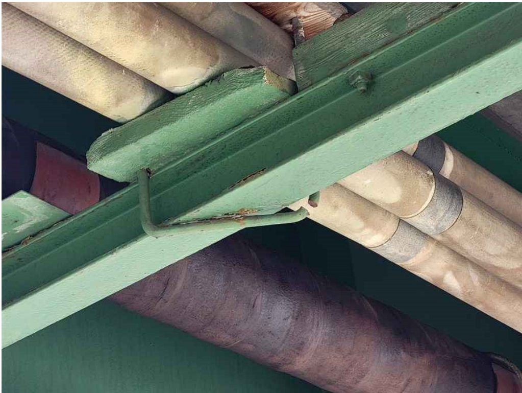
Photo 26: Span 2, Bay 1, the third utility bracket from the North Abutment has a broken "U" bracket. (Looking South).
