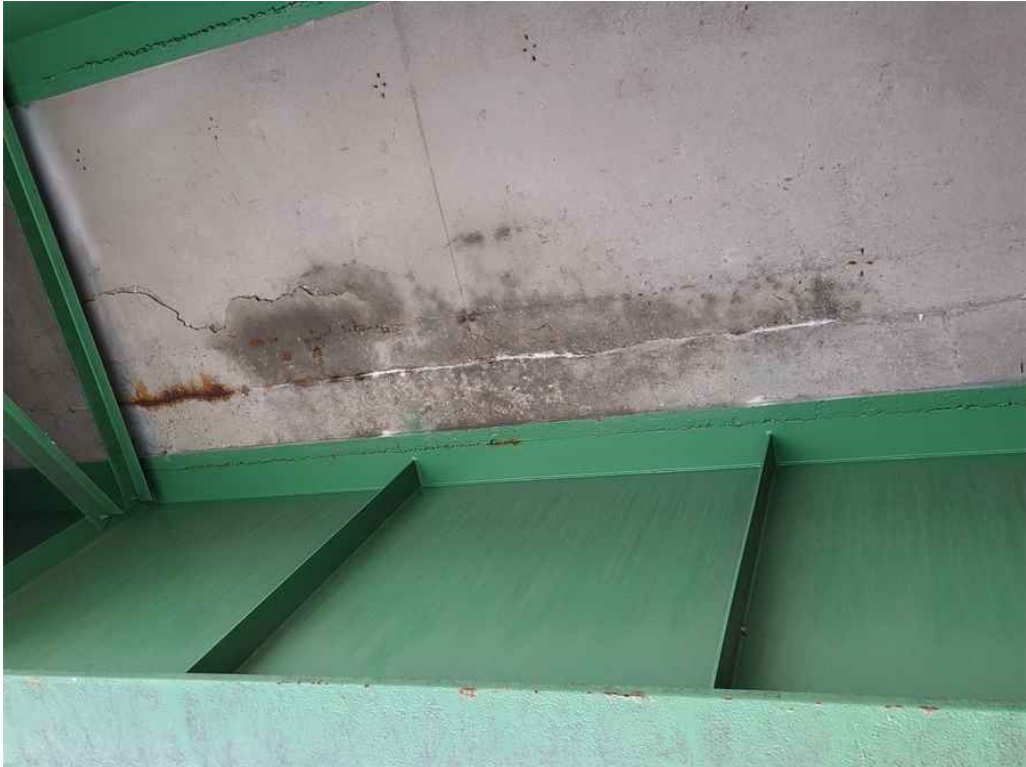
Photo 13: Deck, span 2, bay 4: full length delamination with moderate efflorescence, rust staining and dampness along the longitudinal construction joint.
