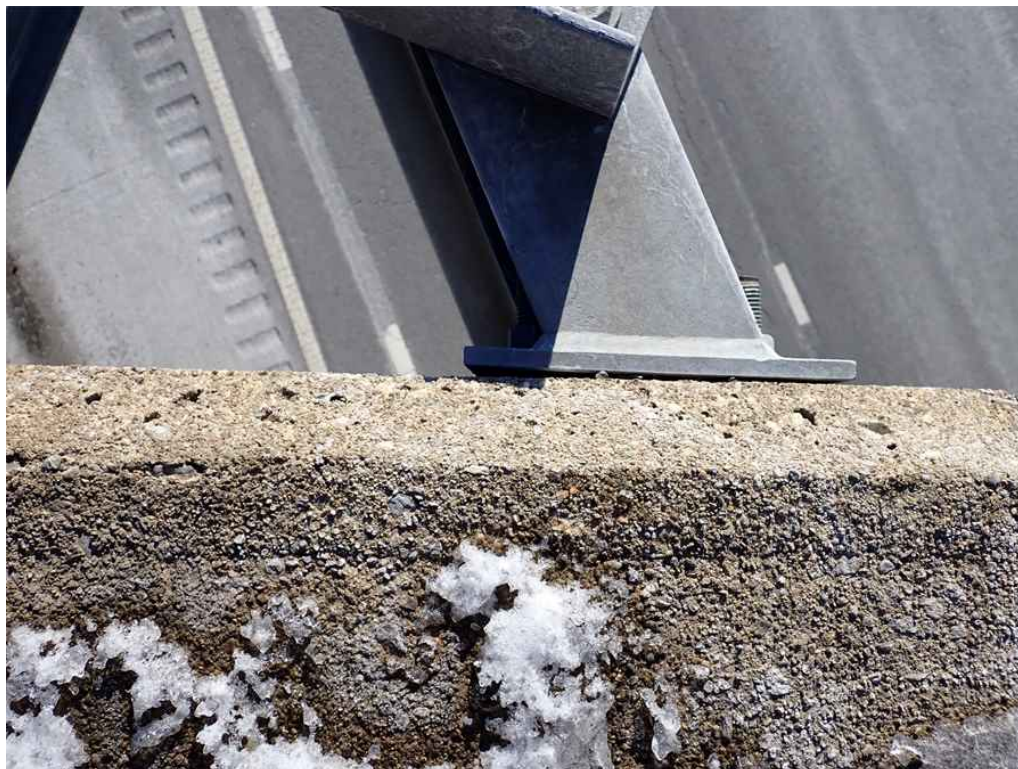
Photo 18: ST-2 westbound overhead sign - Gap between the upper south connection and the sidewalk fascia.
