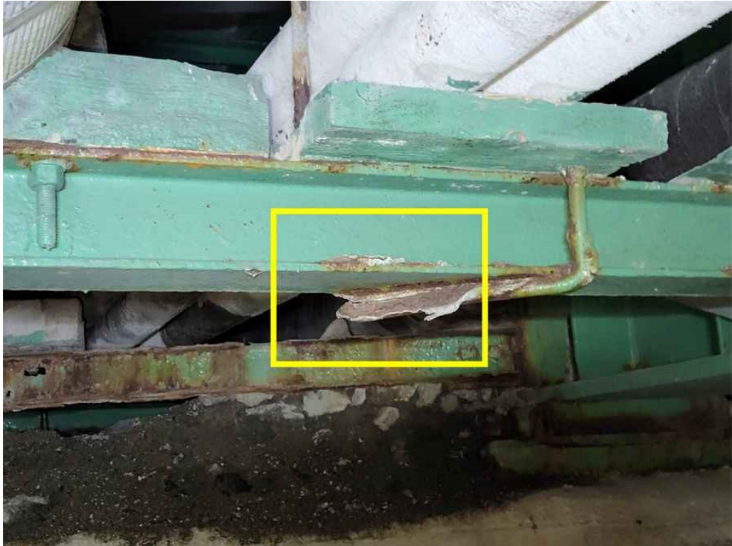
Photo 27: Span 1, Bay 1, the first utility bracket from the pier has rusted with 100% section loss. (Looking North).
