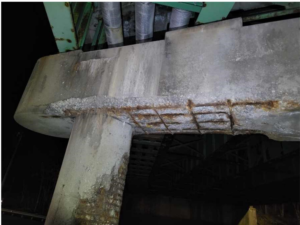
Photo 55: Pier cap, north face, above Column C1: moderate spalling extending into the bottom face with exposed rebar.
