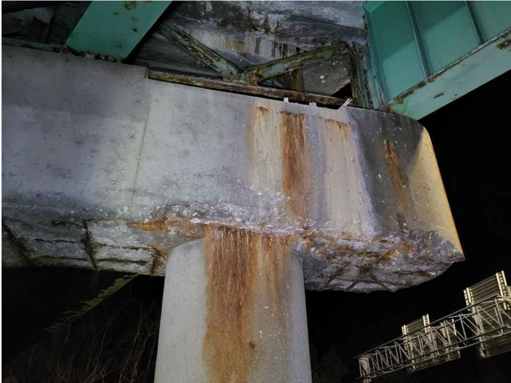
Photo 57: Pier cap, north face, above Column C4: moderate spalling extending into the bottom face with exposed rebar.
