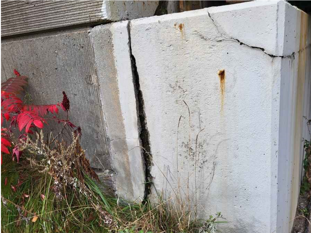
Photo 55: Southeast wingwall: full height vertical crack, up to 3" wide.
