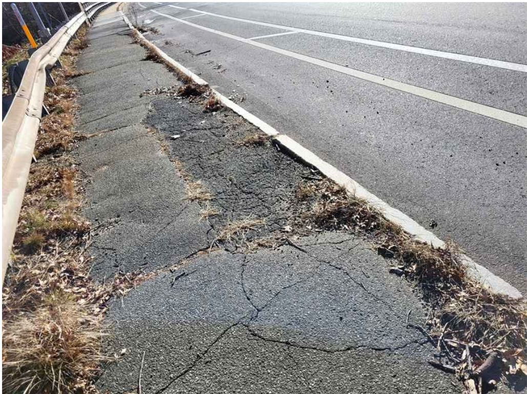
Photo 24: Northeast approach sidewalk: displaced curb sections, several longitudinal and transverse cracks, areas of settlement up to 3" deep throughout. (Looking South).
