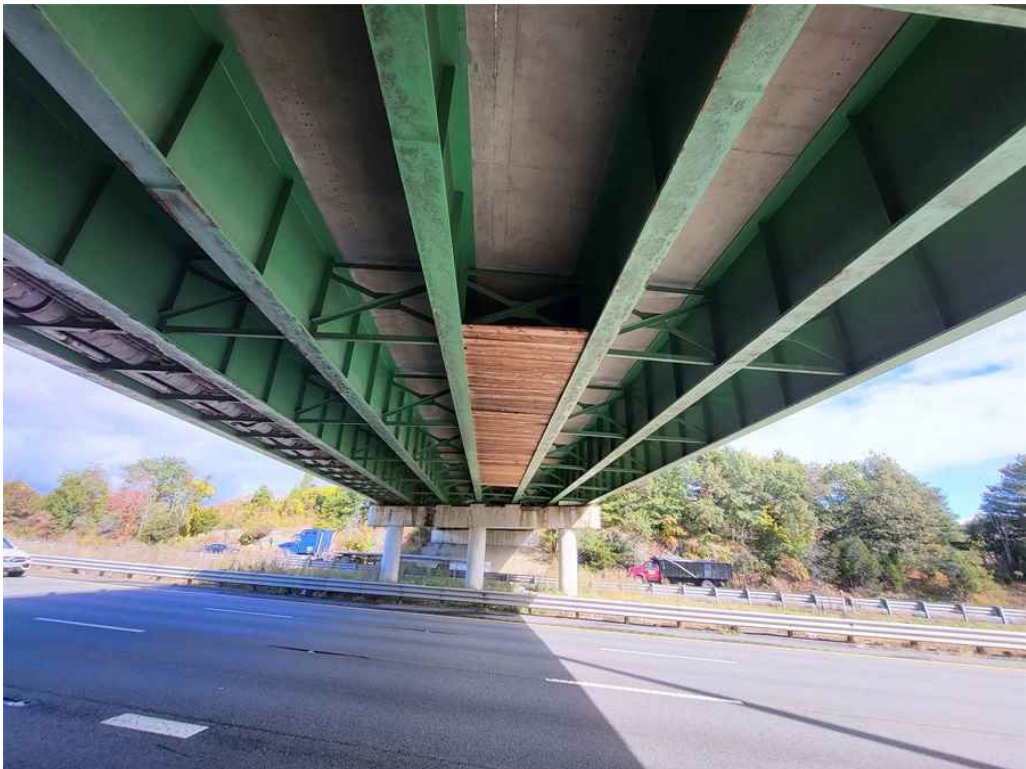
Photo 8: Deck, span 1: bay 4 shielded over the eastbound roadway over the left three travel lanes. (Looking North).
