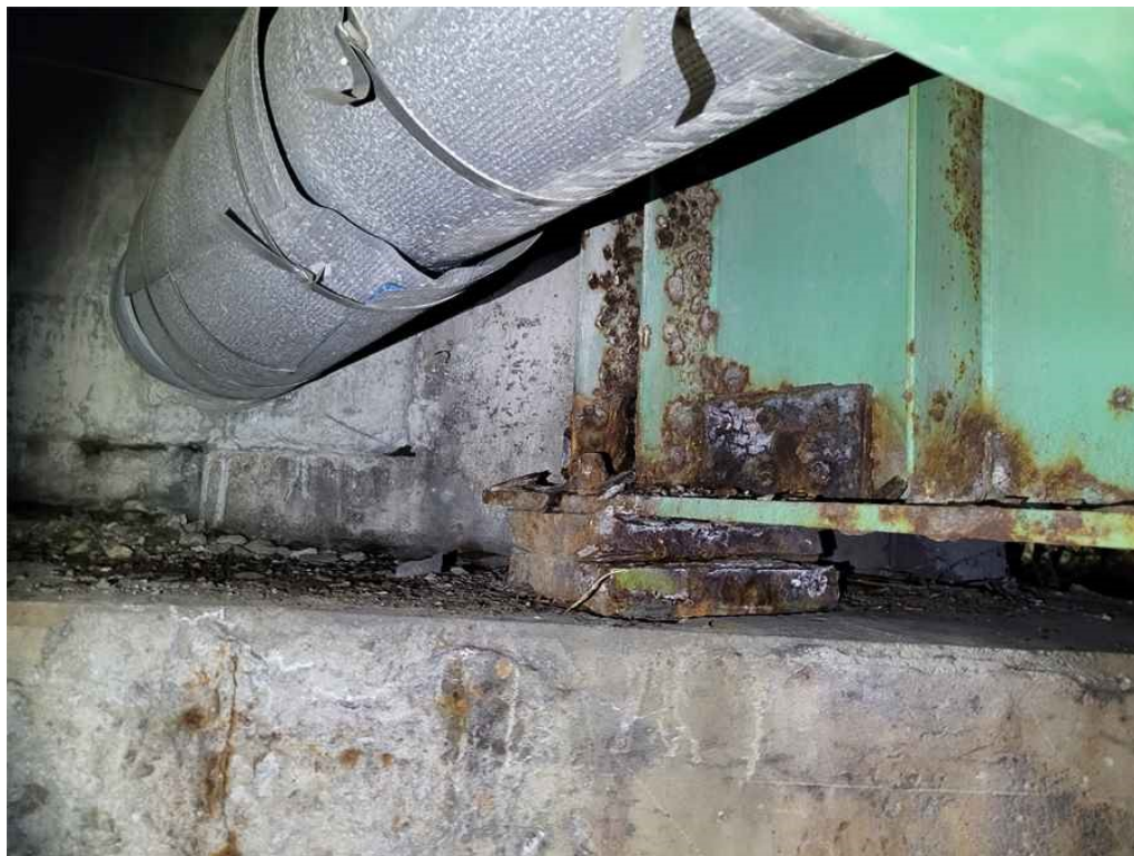
Photo 30: Girder 1: repair plates to the lower web and bearing stiffeners at the north abutment bearing with heavy rusting and minor steel delamination. Also note bearing rust. (West face shown).
