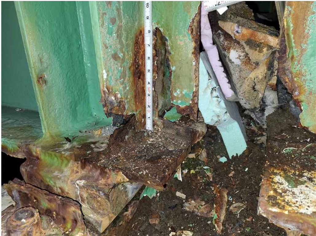
Photo 37: Beam 7: area of 100% section loss at the north end of the web beyond the bearings measuring 7" high x 4" wide at the bottom. Also note the 100% section loss to the stiffener 3" high x 2" wide.
