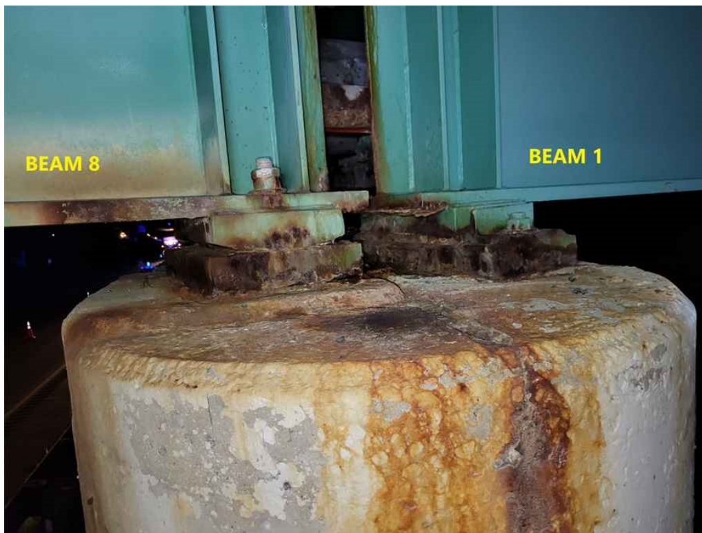
Photo 43: Bearings: moderate rust, lamination and active water leaking from deck joints. Also note west anchor of beam 8 is bent towards North. (Bearing of beams 1 & 8 at pier shown).
