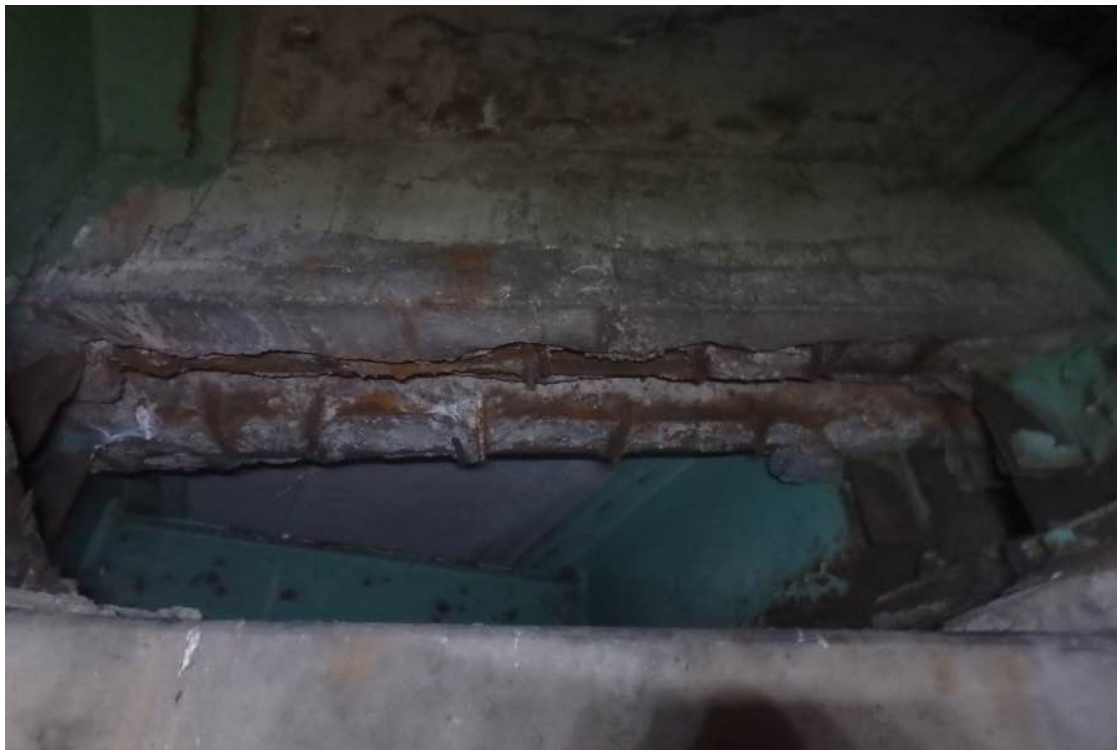
Photo 29: Typical concrete end diaphragm spalling; view at pier.
