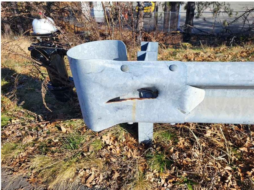
Photo 66: Tear at the northeast guardrail end.
