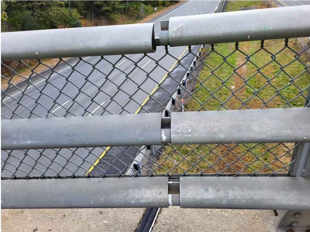
Photo 23: East railing, the top rail is disconnected at the joint over the pier.
