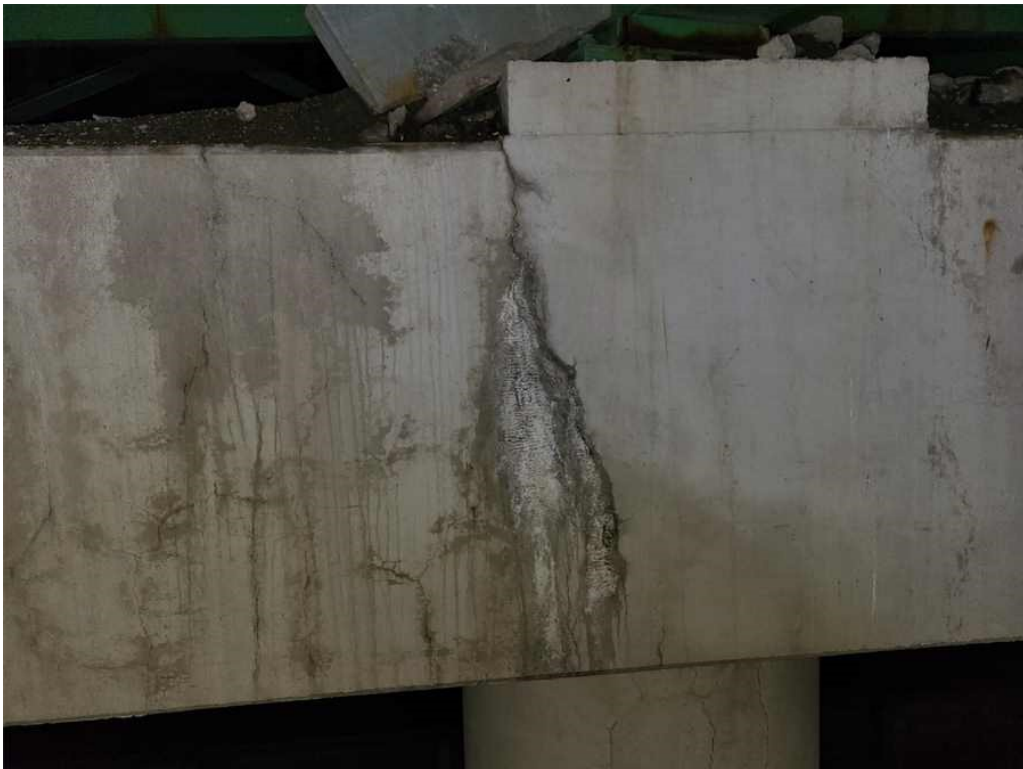
Photo 60: Pier cap, west face, under beam 4, full height vertical crack with light efflorescence, up to 1/8" wide and several hairline map cracking throughout bay 3.
