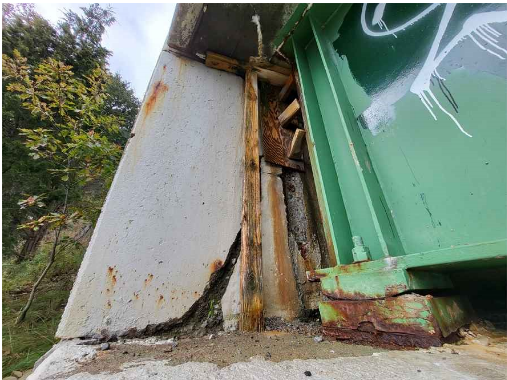
Photo 50: South backwall, behind Beam 7: active leakage, formwork left in place, vertical crack 2" wide x full height and adjacent spall 6" wide x full height x 3" deep with exposed rebar.
