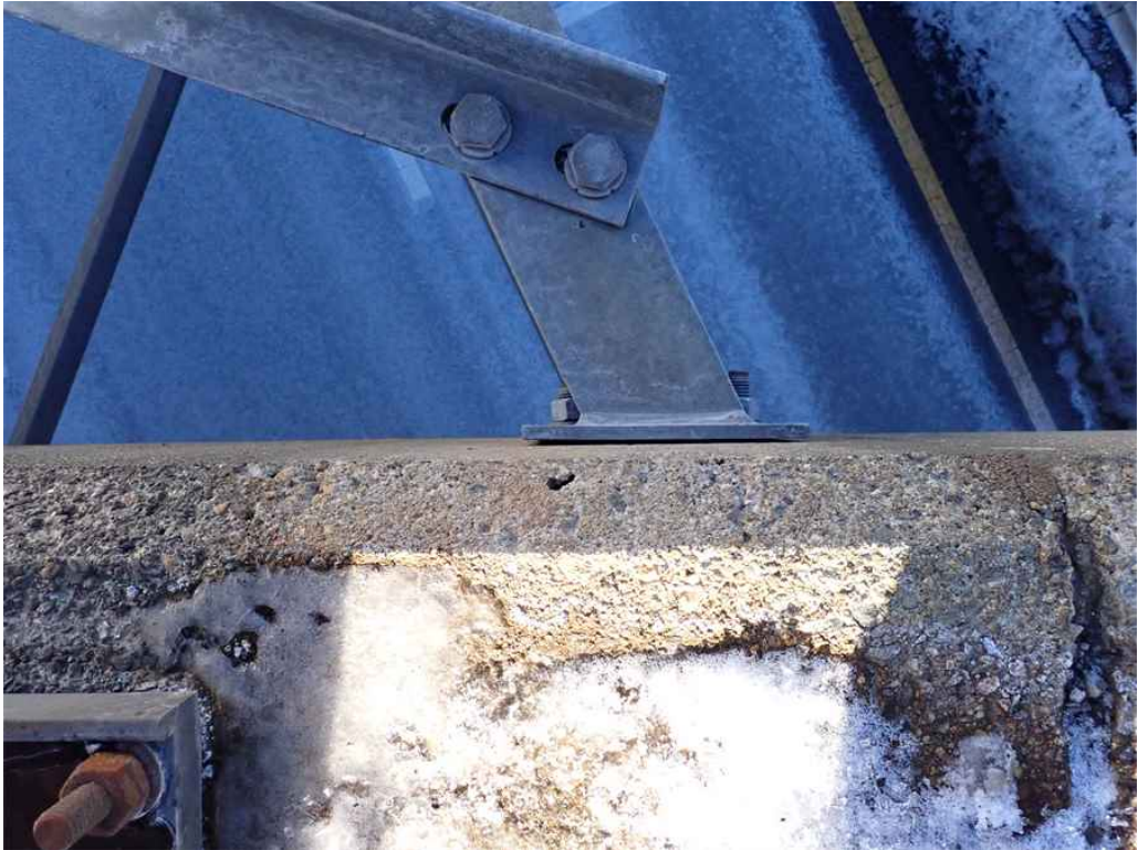
Photo 19: ST-2 eastbound overhead sign - Gap between the upper north connection and the sidewalk fascia.
