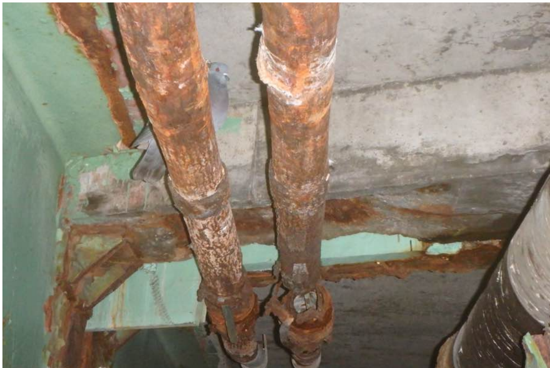
Photo 19: Bay 10 utility pipe rust at the pier joint.
