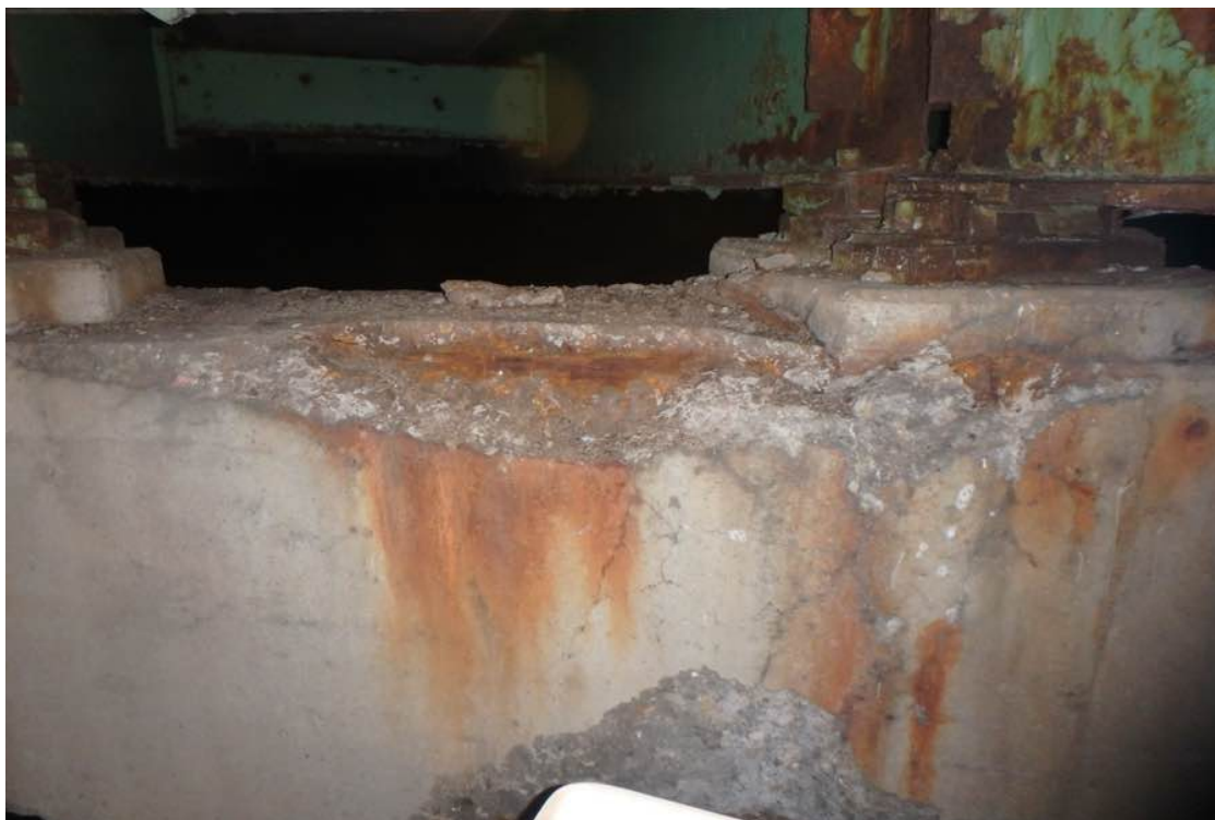
Photo 40: Pier cap, spall between Beams 108 & 109.
