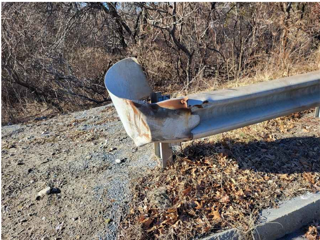
Photo 65: Impact damage at the southwest guardrail ends.
