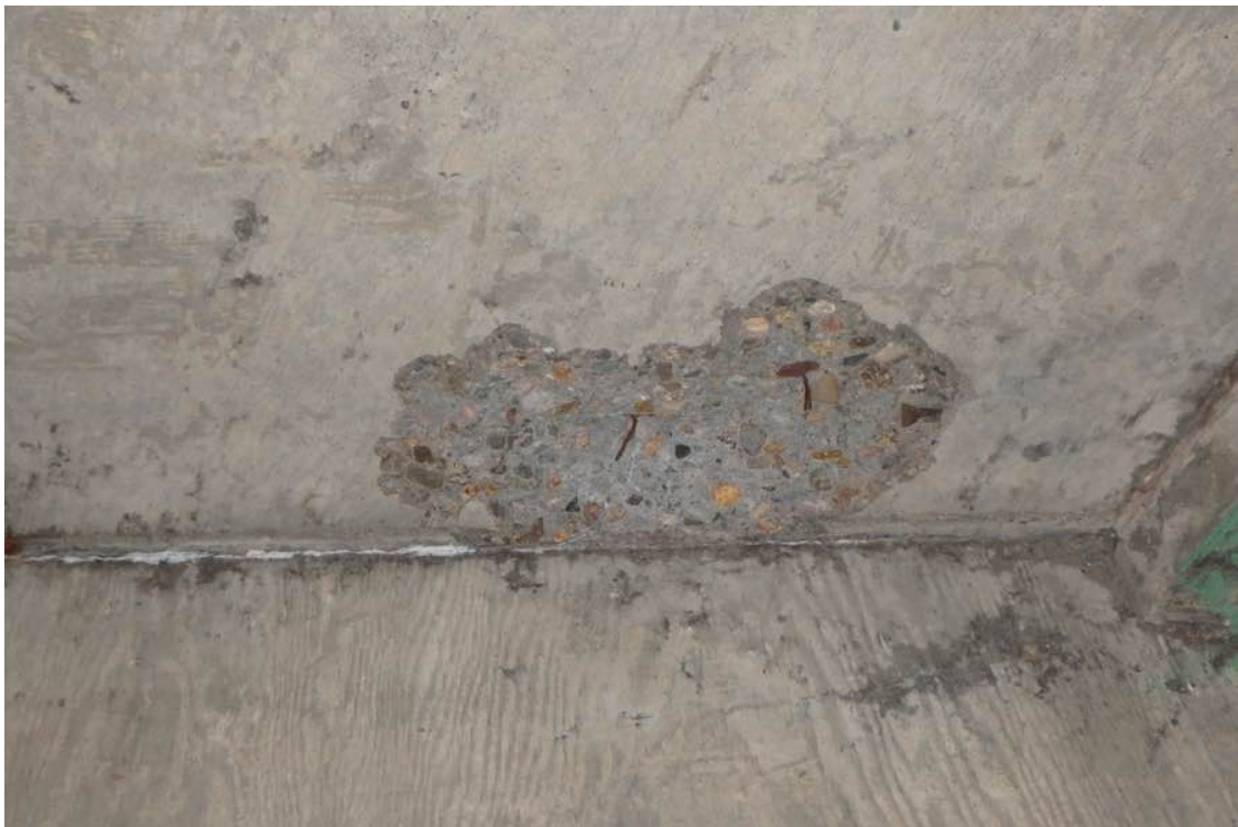
Photo 6: Span 1, Bay 6, spalling at the north end.
