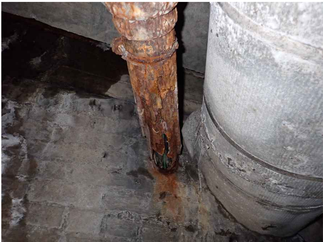
Photo 12: Severe laminar rust and section loss to the steel conduit in Bay 12 of Span 2 at the backwall.
