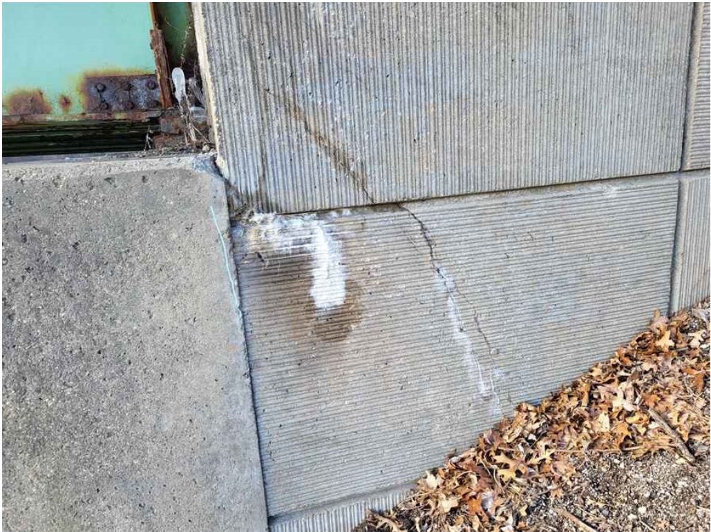
Photo 45: Northeast wingwall: cracks with efflorescence at the abutment and a long narrow diagonal crack extending from the bridge seat/backwall area. (Looking West).
