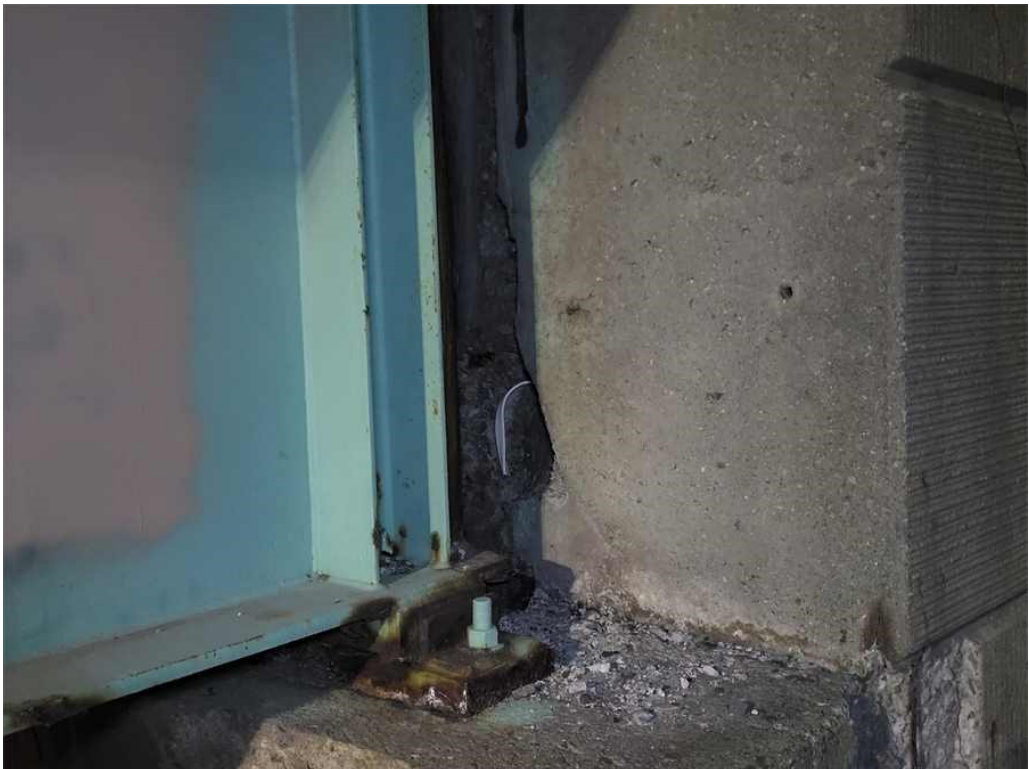
Photo 42: South backwall, bay 12: Spall behind Girder 14, full height x up to 1.0' wide x 5" deep.
