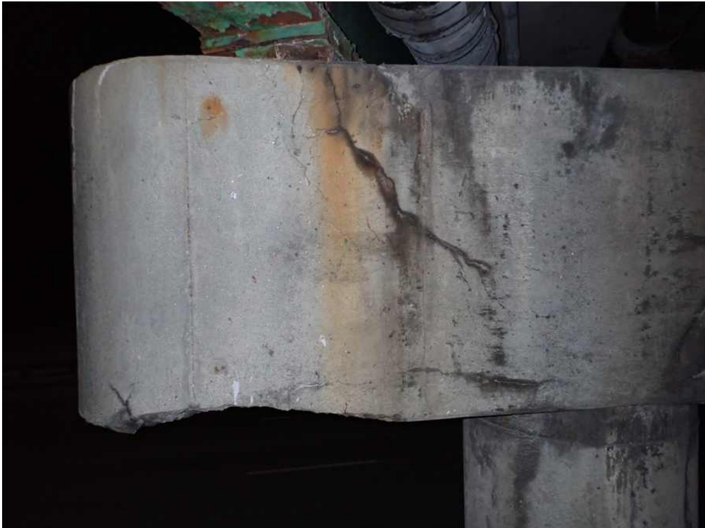
Photo 46: Pier cap, north face, east end with diagonal crack.
