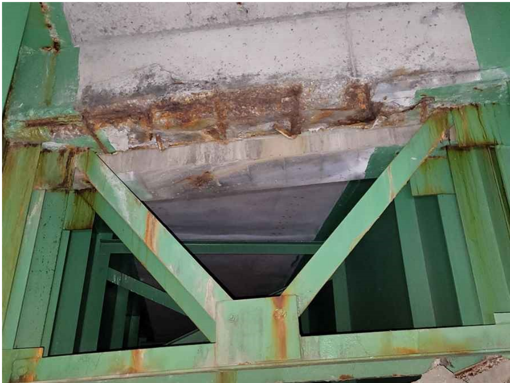
Photo 46: Concrete diaphragms at the Pier: moderate/severe spalling and delamination, full bay length x full width x 3" deep with exposed and rusted rebar, typical. (Bay 2, span 2 shown).
