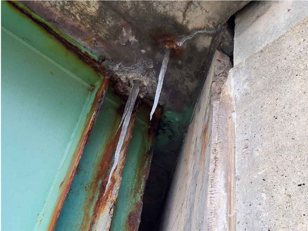
Photo 5: Span 1, east overhang: minor spall around the north end weep-hole. Also note the frozen and clogged deck weeps.
