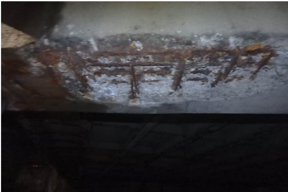
Photo 42: Pier cap, spall between Columns 1 & 2.
