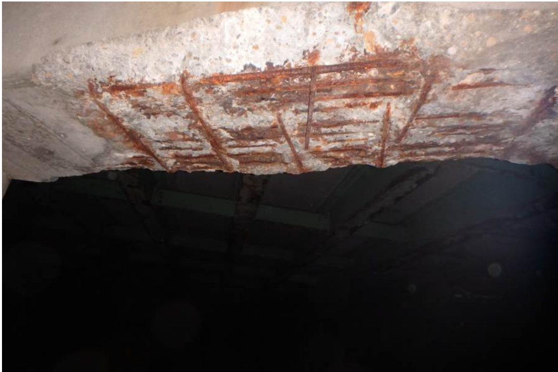
Photo 45: Pier cap, spall between Columns 4 & 5.
