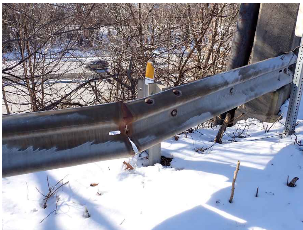
Photo 48: Northeast approach guardrail with broken weld.
