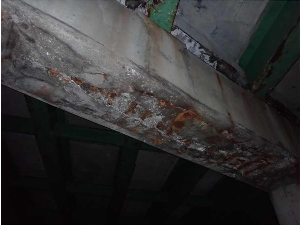
Photo 39: Pier cap underside between Columns 4 and 5 with spall and exposed rusted rebar.
