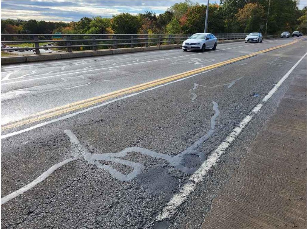
Photo 1: Wearing surface: several random longitudinal sealed and non-sealed cracks and a few patched potholes throughout. (Span 2 shown, Looking South).
