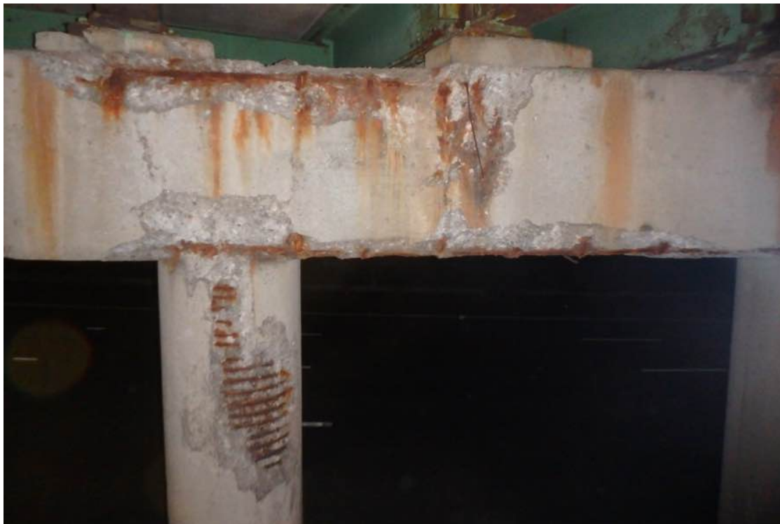
Photo 39: Pier pedestal for Beam 103 has spalling on the southwest corner. Note the spalling in the south face of the cap and Column 2.
