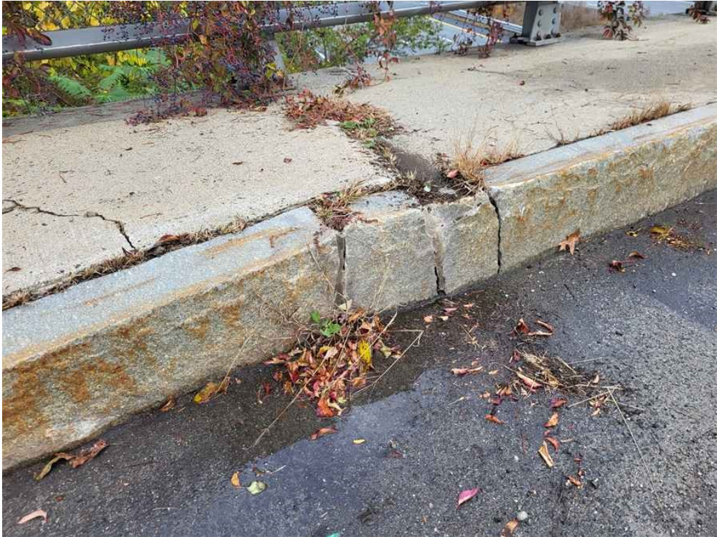
Photo 17: West curb, at south deck joint, granite section has full height cracks, up to 1/2" wide.
