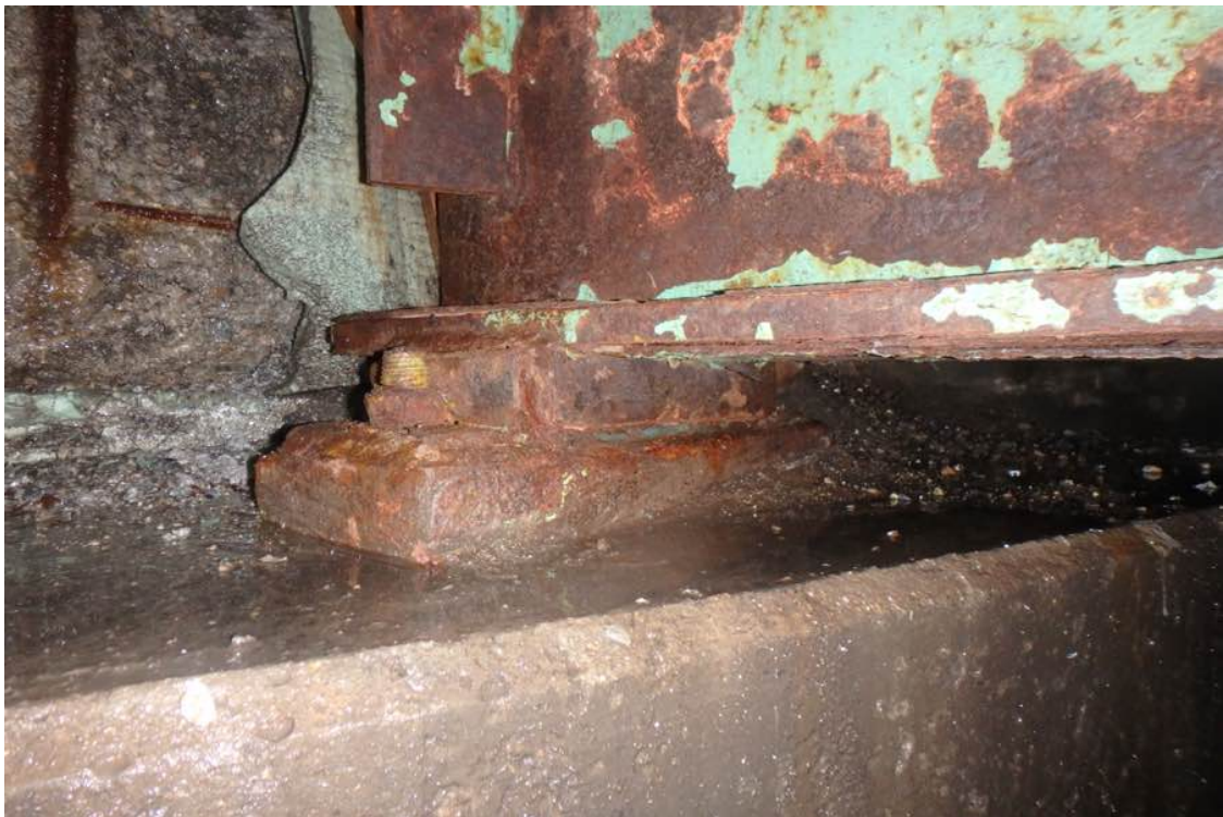
Photo 28: Typical rust throughout all bearings; view at north abutment.
