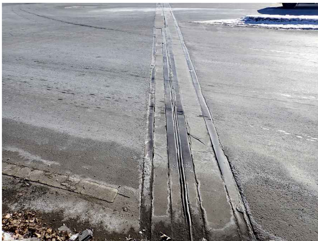
Photo 16: North Abutment joint in the southbound lanes.
