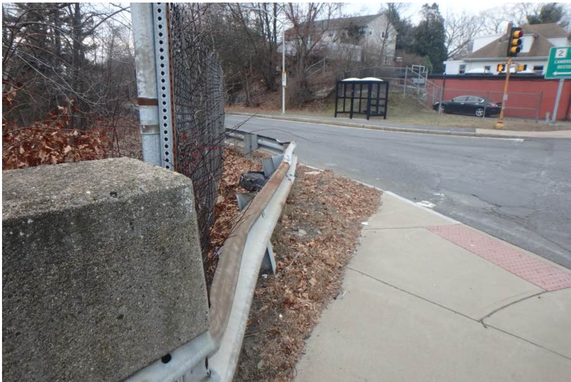
Photo 54: Southeast approach rail damage.
