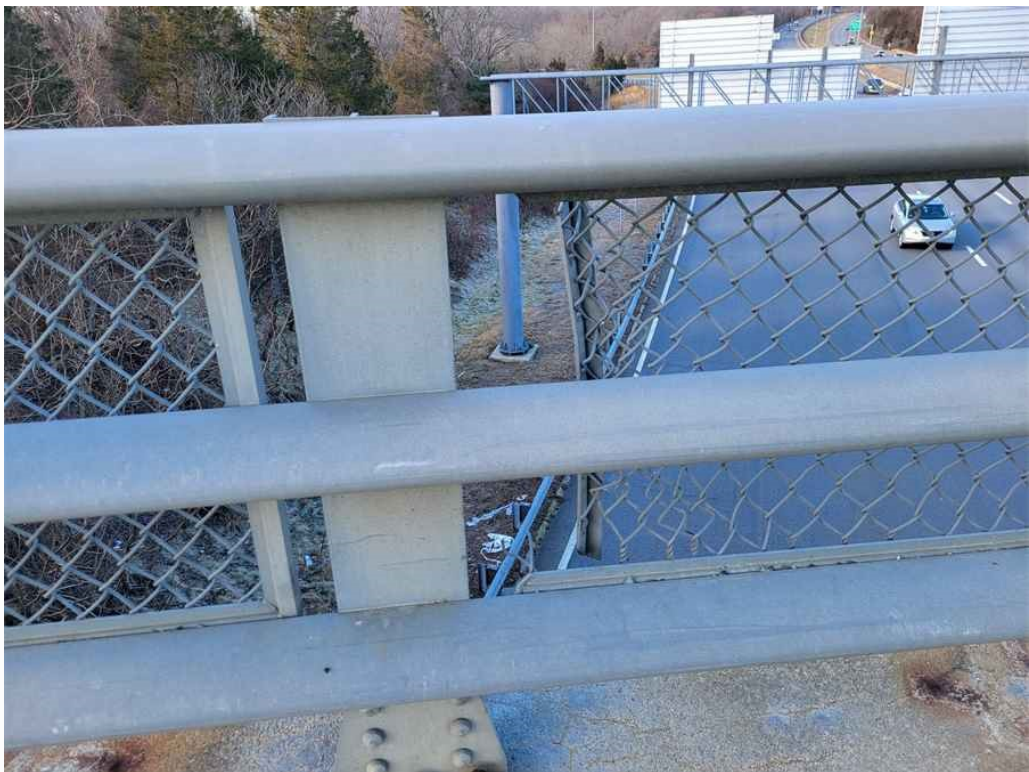
Photo 19: Safety fence along the west bridge rail: area of disconnection (gap) near the south end.
