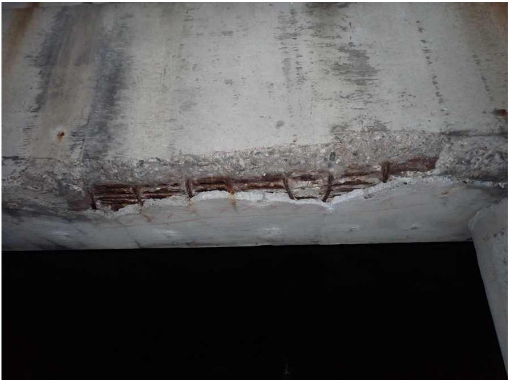
Photo 38: Pier cap underside, north edge, between Columns 3 and 4 with spall, exposed rebar and delamination to the old repair.
