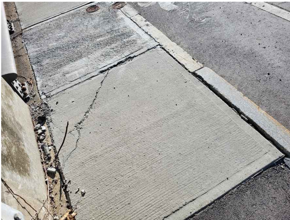
Photo 25: Diagonal crack in the northeast concrete approach sidewalk, 3.5' long x 1/8" wide. Also note the displaced curb section.
