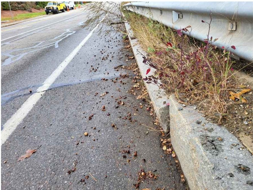
Photo 16: Curb at northeast corner is leaning into the roadway, up to 3". (Looking north).
