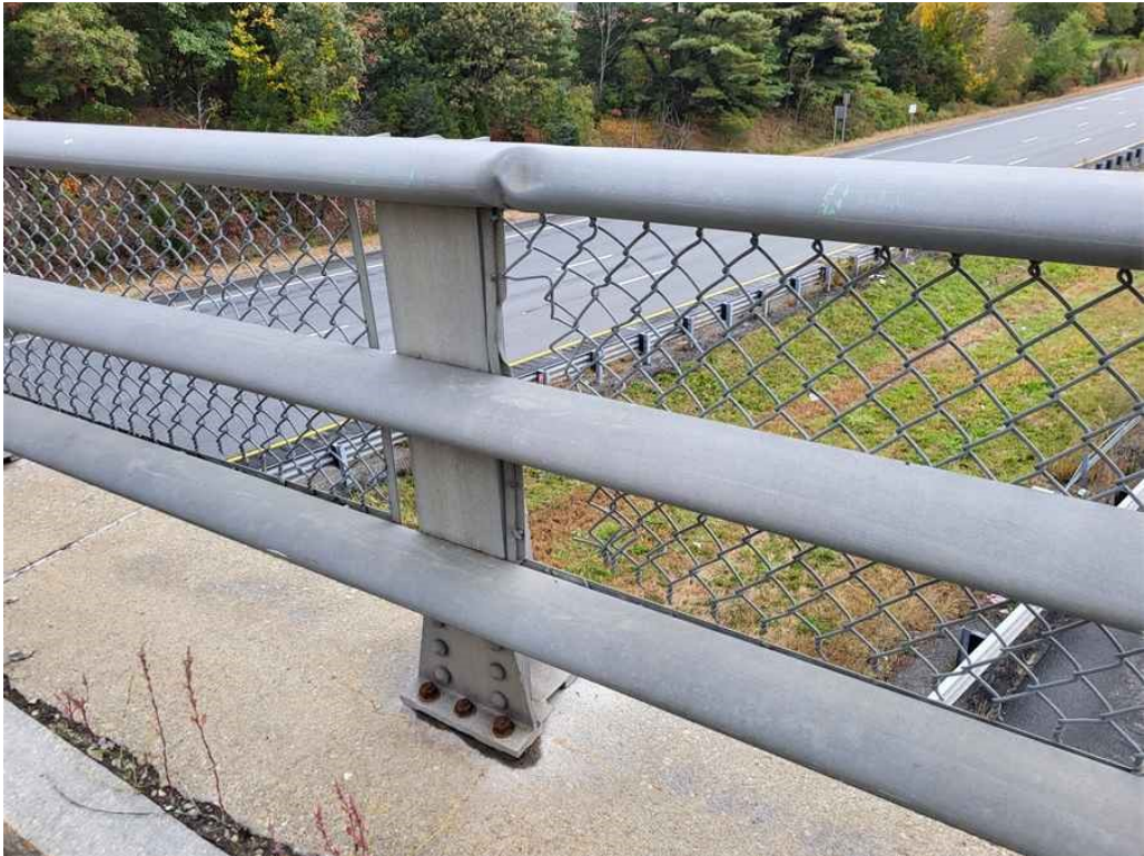
Photo 22: Several random minor dents along the top hand rail on the east railing. Also note the detached metal fencing. (Post #16 from south shown)
