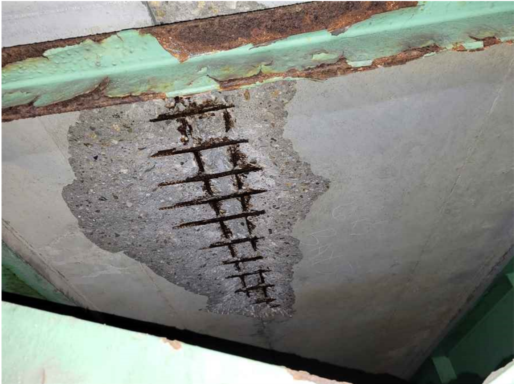
Photo 8: Deck, span 1, bay 2: at cross frame 6, spalling and delamination, up to 7' long x 3.5' wide x up to 3" deep, with exposed rebar.
