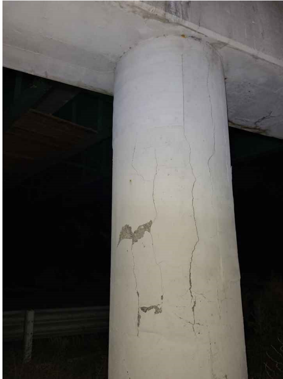
Photo 67: Column 2: nine (9) full height vertical cracks up to 1/4" wide, hollow area at the top half and a spall at the west face, 15" wide x 5" high x 1.5" deep.
