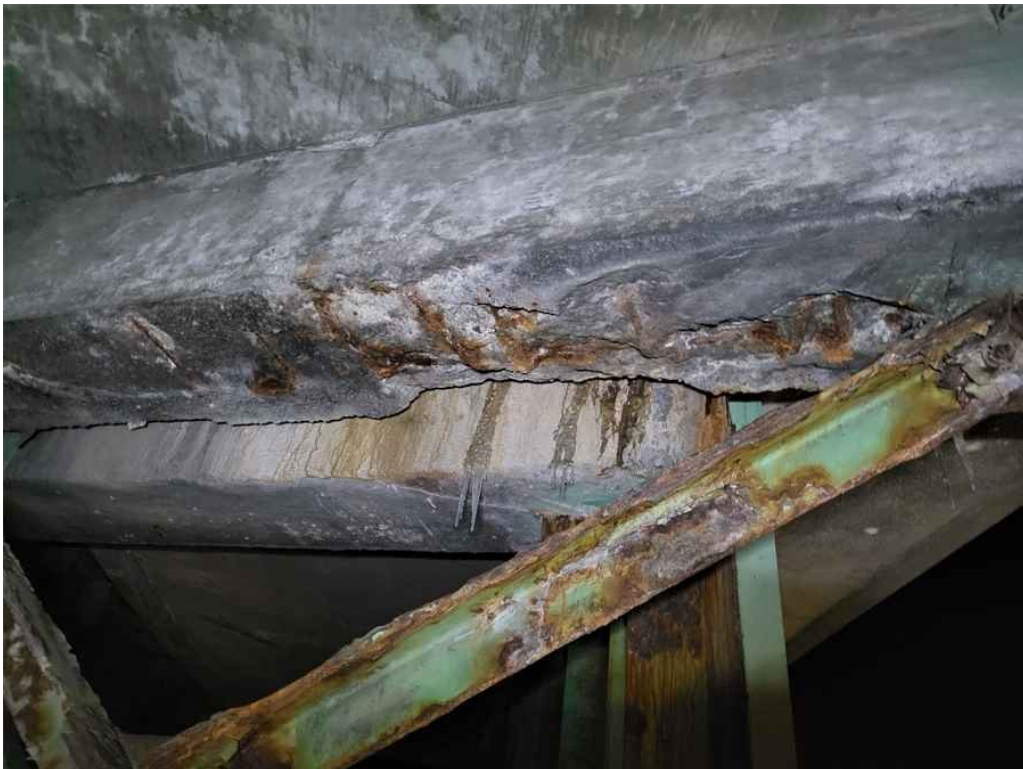
Photo 38: Span 1, bay 6 diaphragm encasement at the pier: full length delamination, rust stains, 18" L x full width x 1.5" D spall with exposed rebar. Also notes steel cross frames peeling paint & rusting.
