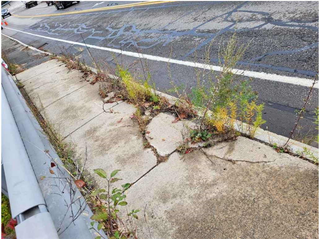
Photo 33: Northwest approach sidewalk: several concrete pads are cracked at the east corners, up to 1" wide with moderate vegetation growth. (Looking North).
