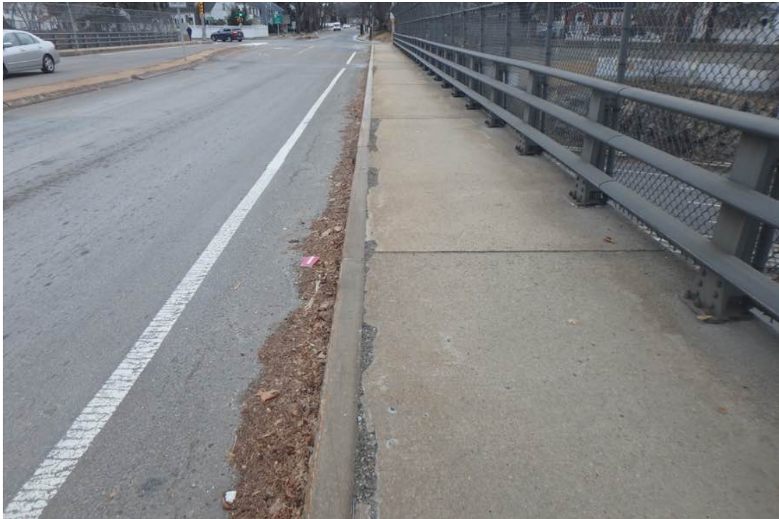
Photo 16: Typical sidewalk spalling along the curb joint.
