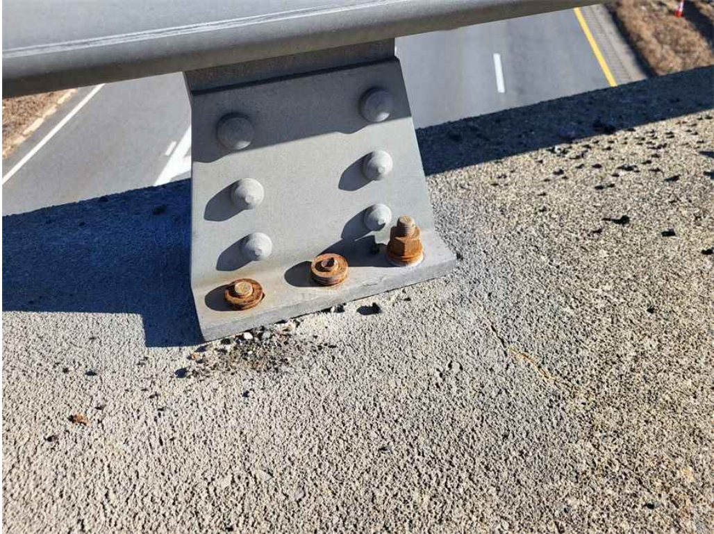
Photo 16: East railing: missing anchor bolt nuts at post #31.
