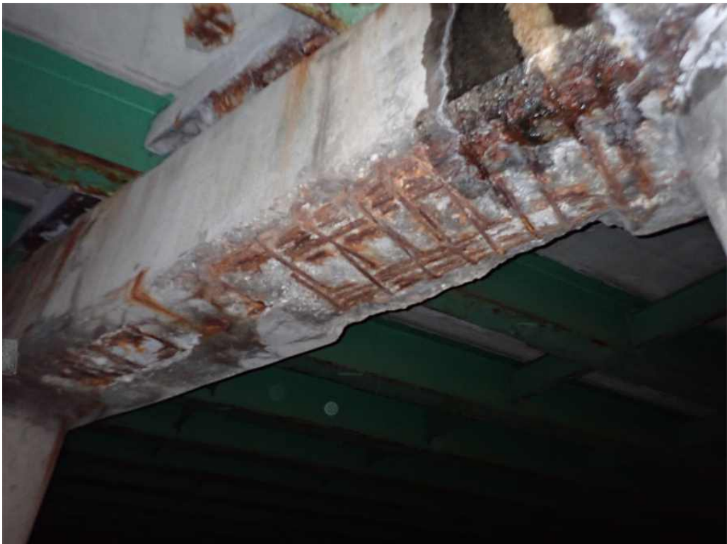
Photo 40: Pier cap underside between Columns 5 and 6 with spall and exposed rebar.
