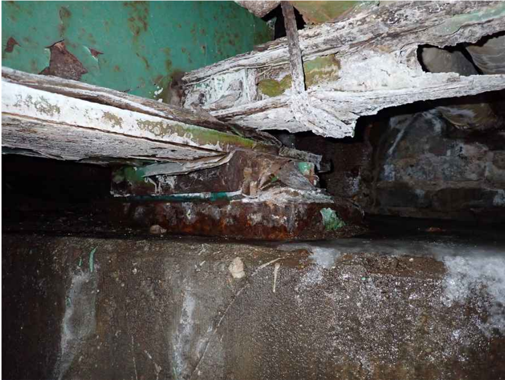
Photo 25: Typical rusting to the abutment bearings with moderate laminar rust.
