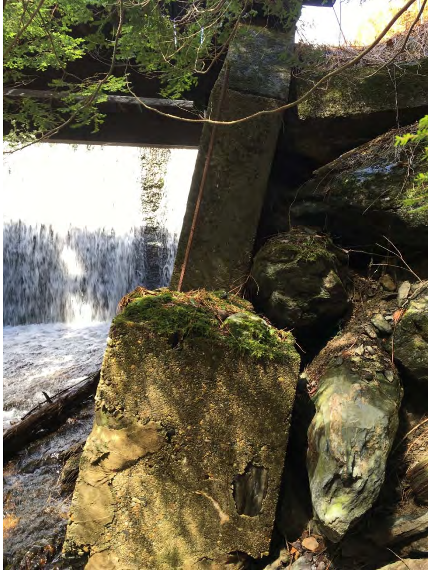
Figure 4. Left concrete training wall slipped off of its foundation and resting on concrete apron
