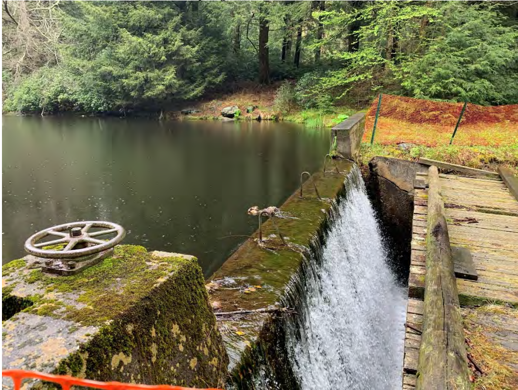
Looking across Becker Pond Dam at the spillway and the wooden bridge. The orange fencing is in place due to the unsafe condition of the abutments and the bridge.
