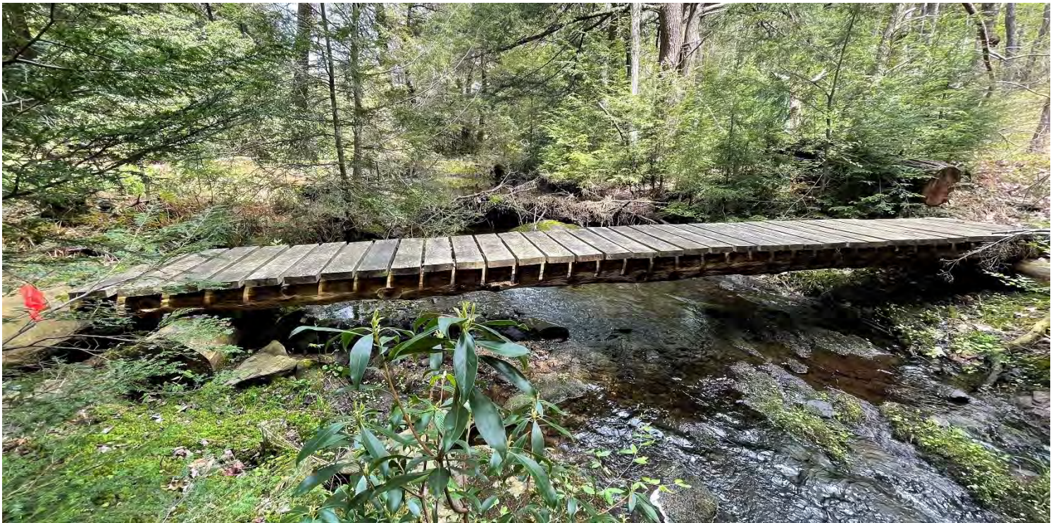
Photo #2: View of the existing footbridge, upstream of Becker Pond Dam. This bridge will remain in place, providing access across the stream.
