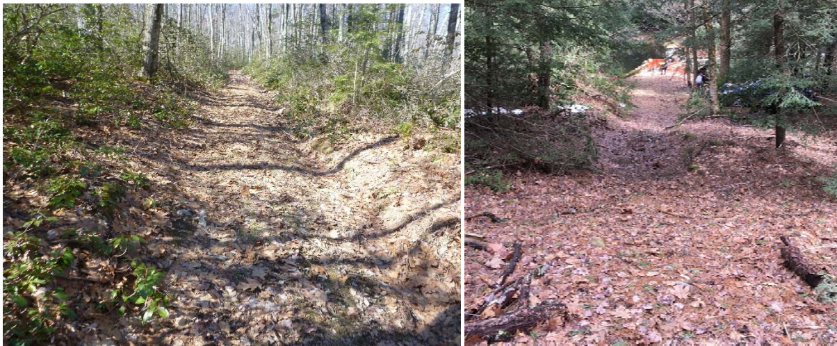
Figure 11. Existing dirt access road to be used during the removal of Becker Pond Dam (left) looking north along the road and (right) looking east towards the dam.
