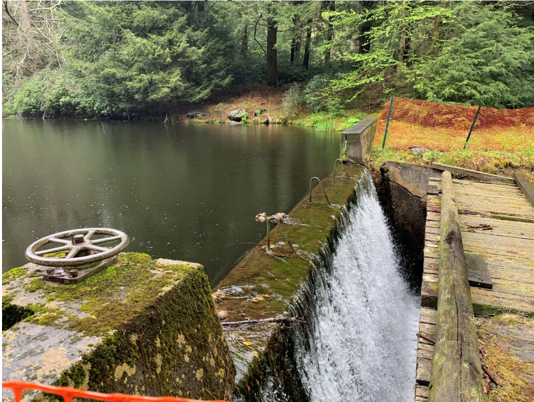
Looking across Becker Pond Dam at the spillway and the wooden bridge. The orange fencing is in place due to the unsafe condition of the abutments and the bridge.
