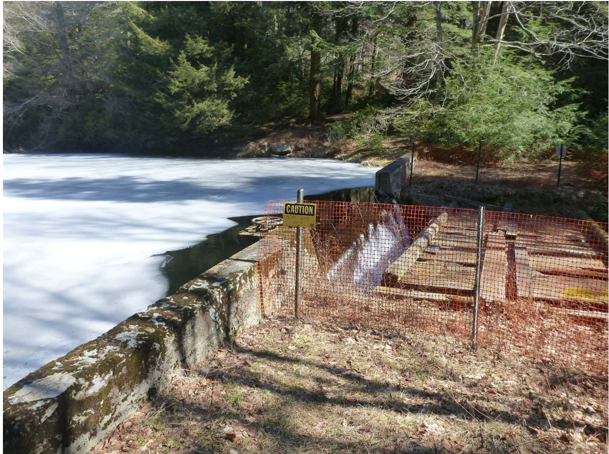
Figure 2. Becker Pond Dam showing concrete core wall, spillway, and failing bridge
