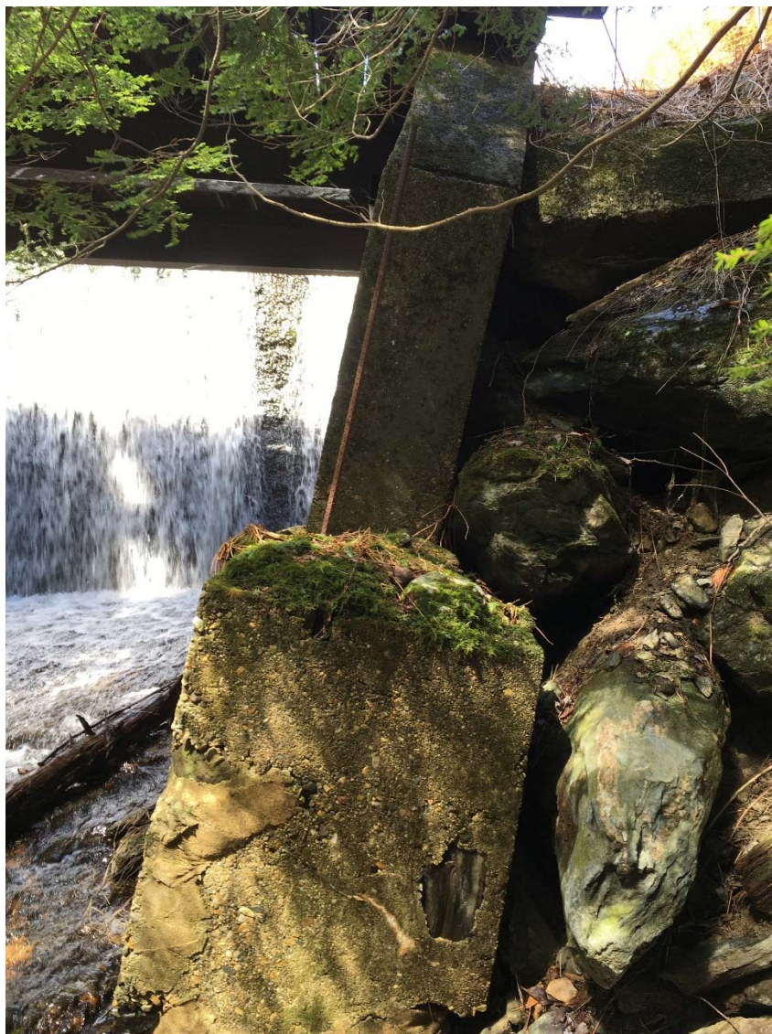
Figure 4. Left concrete training wall slipped off of its foundation and resting on concrete apron
