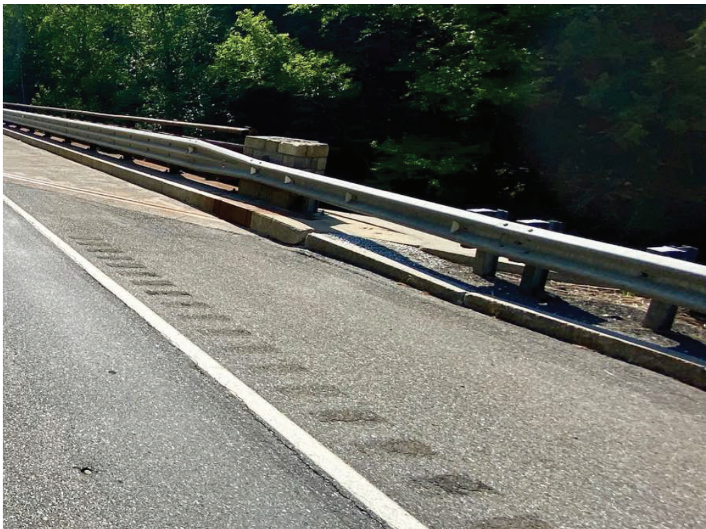
Photo 26: Guardrail posts improperly spaced at southwest guardrail transition.
