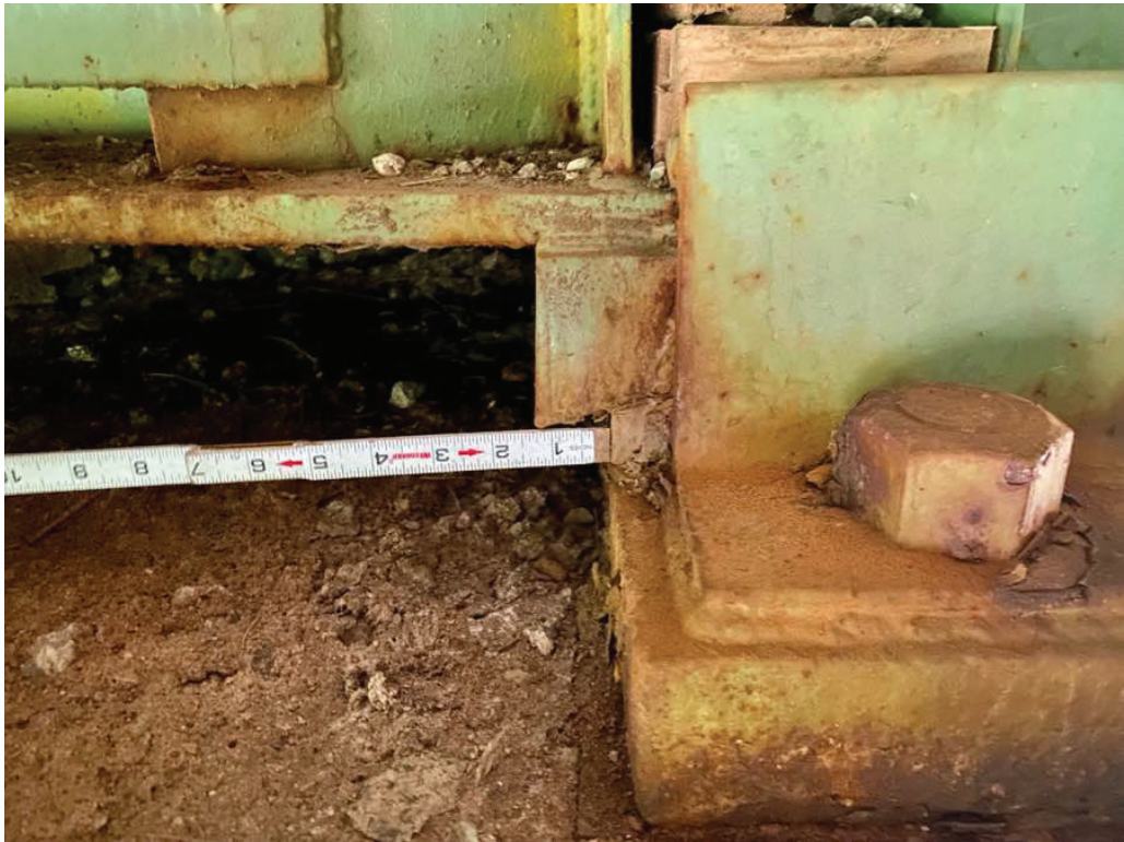
Photo 15: Bearing overexpanded, girder 5 bearing at west abutment.
