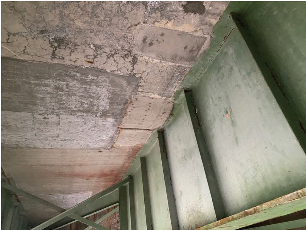
Photo 4: Bay 2, overfilled concrete patches. Typical.
