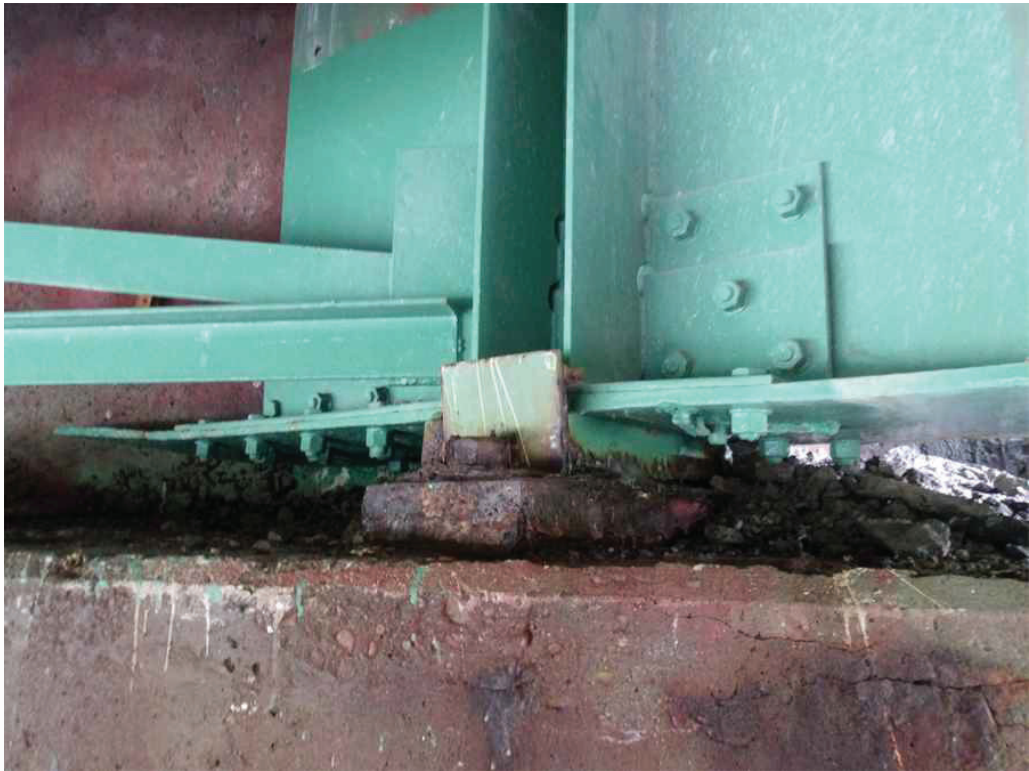
Photo 23: South side of Girder 1 and the bearing at the West Abutment, looking northwest. Note the bent bottom flange, missing bottom flange repair nut, and rusted bearing.
