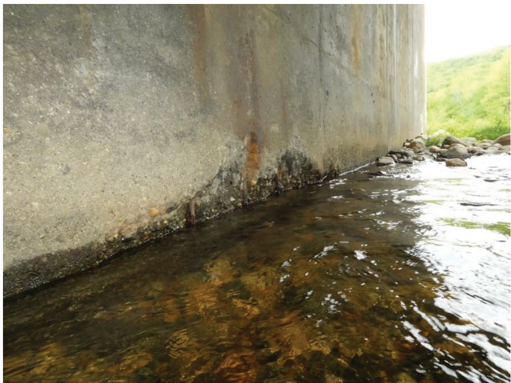
Photo 11: East breastwall, north end, scaling along the waterline.
