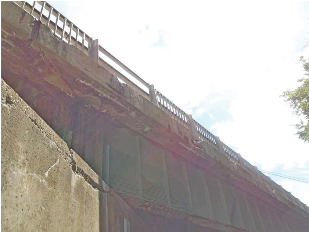
Photo 10: Underside of the South Deck Overhang in the East Span, looking northeast. Note the spalls on the deck underside and the vertical face of the safetywalk.
