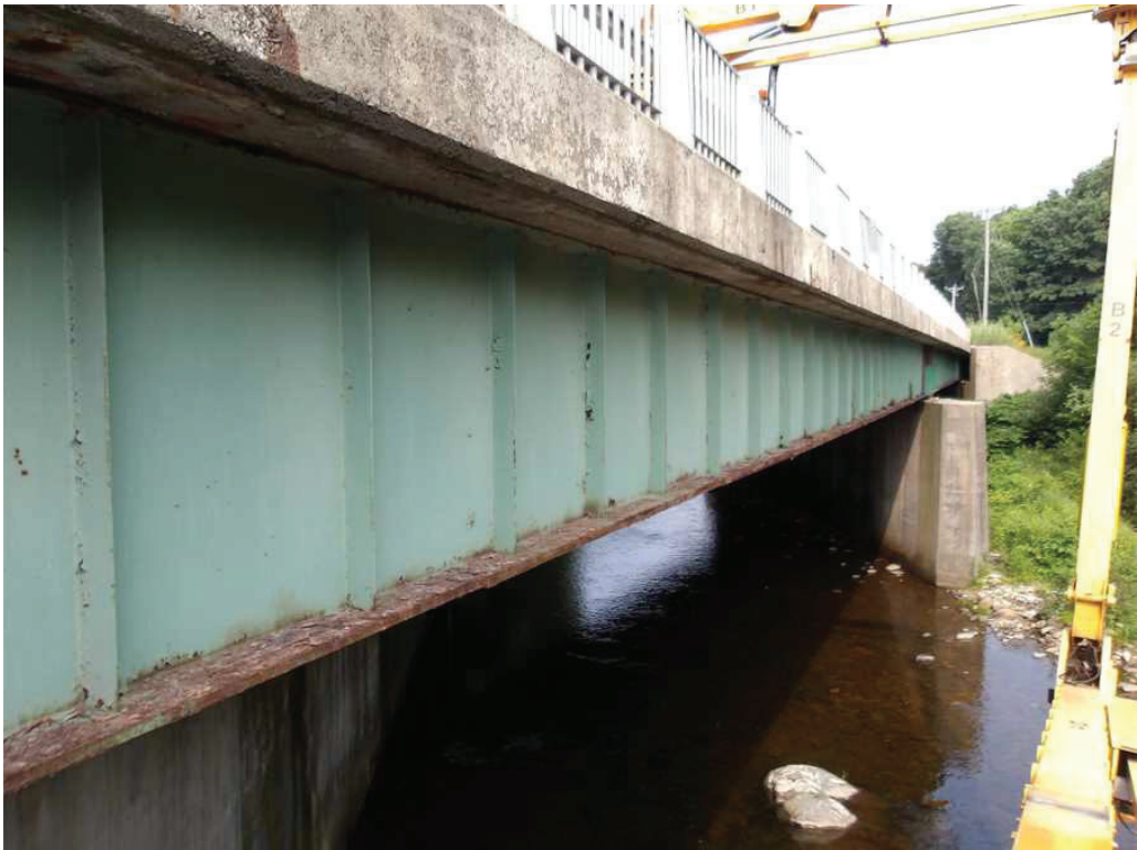
Photo 30: North side of Girder 7, looking southwest. Note the areas of heavy and laminated rust.
