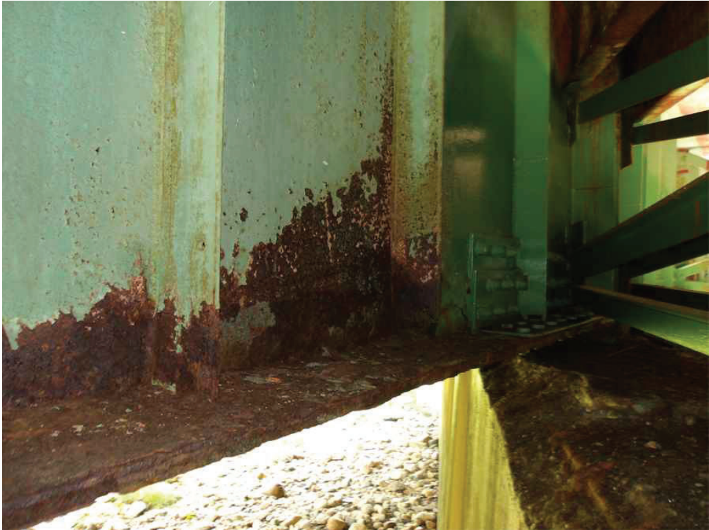
Photo 29: South side of Girder 5 at the Pier, looking northeast. Note the areas of section loss and the stiffener rust hole.
