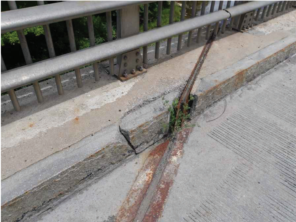
Photo 12: North Curb and Safetywalk at the Pier, looking north. Note the broken curb, vegetation, safetywalk spall, and the rust on the deck joint.
