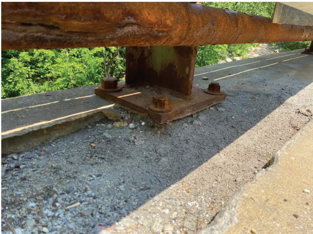
Photo 9: Spall in north rail base, undermining bridge railing post, with two anchor bolts exposed.
