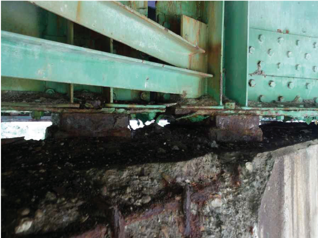
Photo 28: North side of Girders 4 and 10 and the bearings at the Pier, looking southeast. Note the gap between the bottom flange and repair angle for Girder 10 and the rusted bearings.
