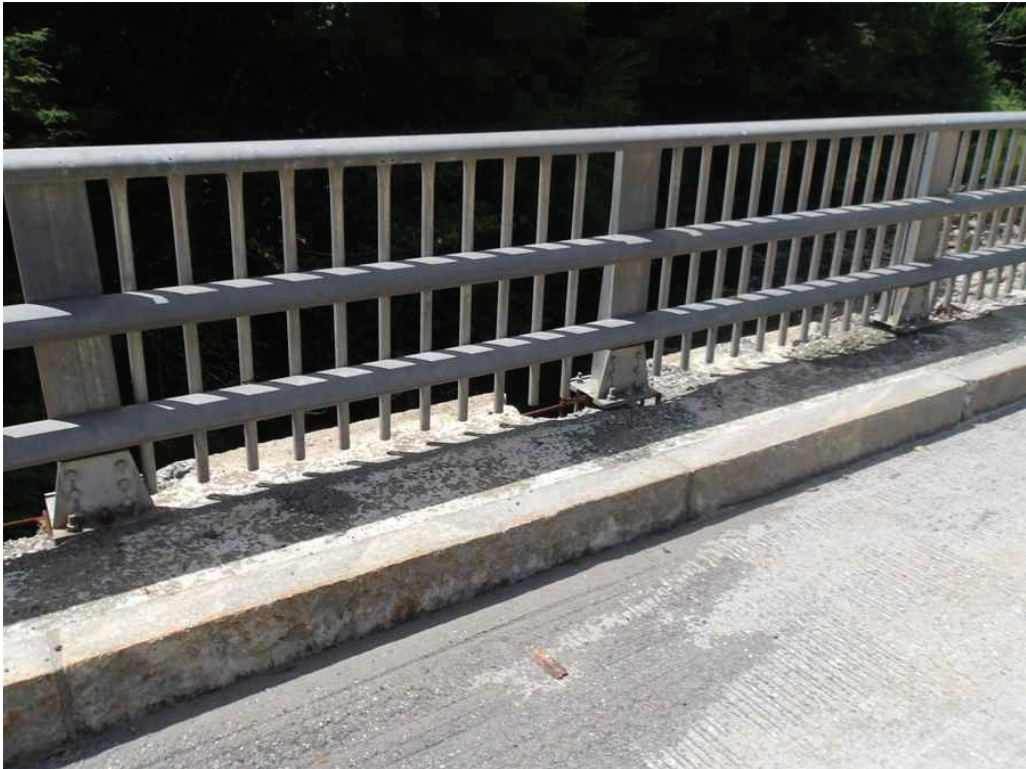
Photo 16: South Safetywalk in the East Span between the third and fifth post from the Pier, looking southwest. Note the spalls and undermined post.
