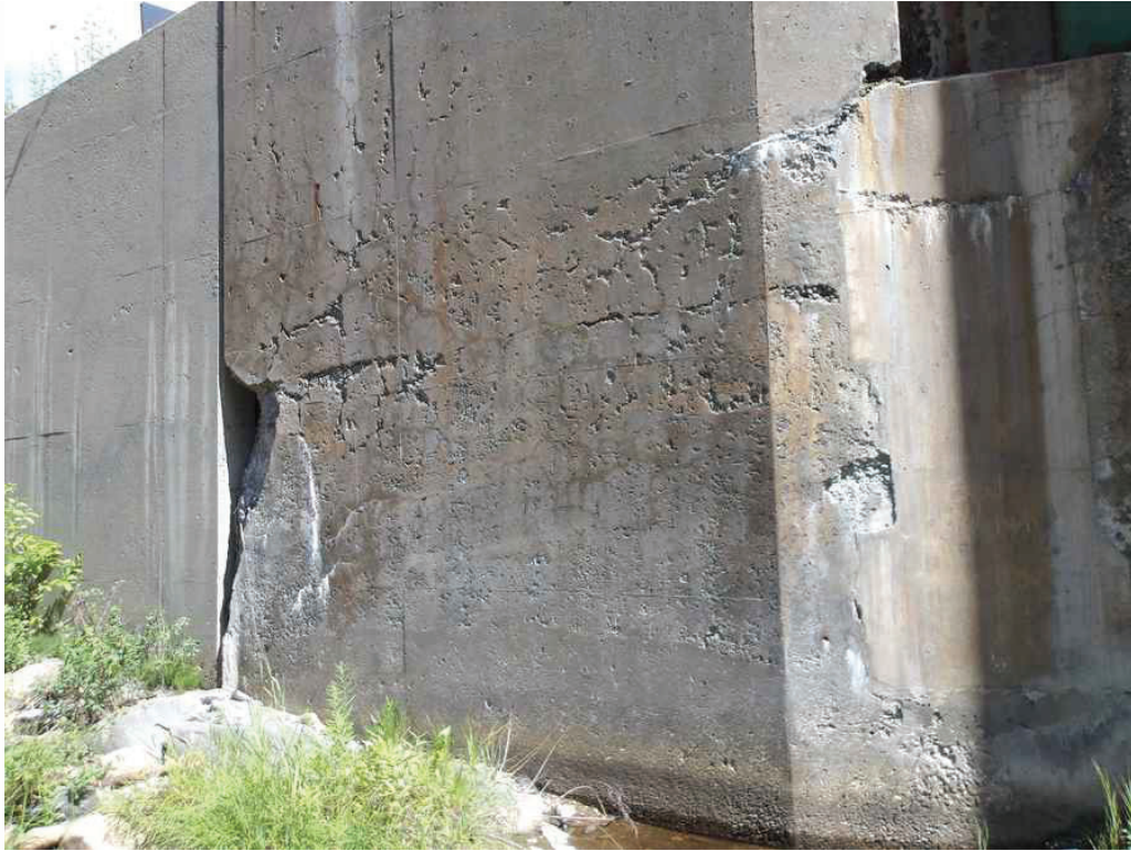
Photo 39: West Abutment at the South Angle Point and the Southwest Wingwall, looking west. Note the spall, scaling, and cracking.
