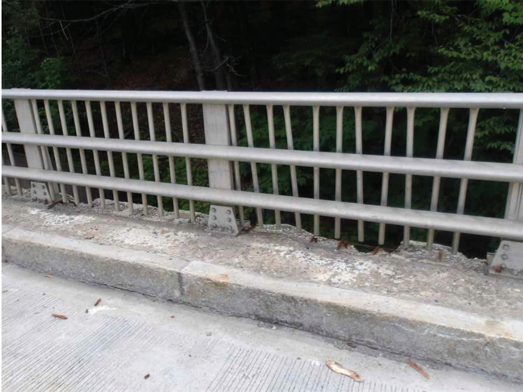
Photo 18: South Safetywalk in the East Span between the twelfth and fourteenth post from the Pier, looking southeast. Note the spalls and undermined posts.
