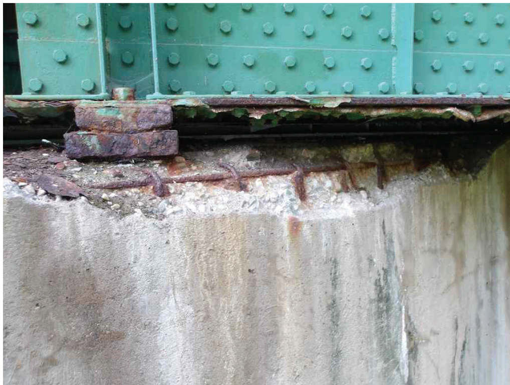
Photo 44: West side of the Pierwall below Girder 1, looking southeast. Note the spall and the undermined and rusted bearing.
