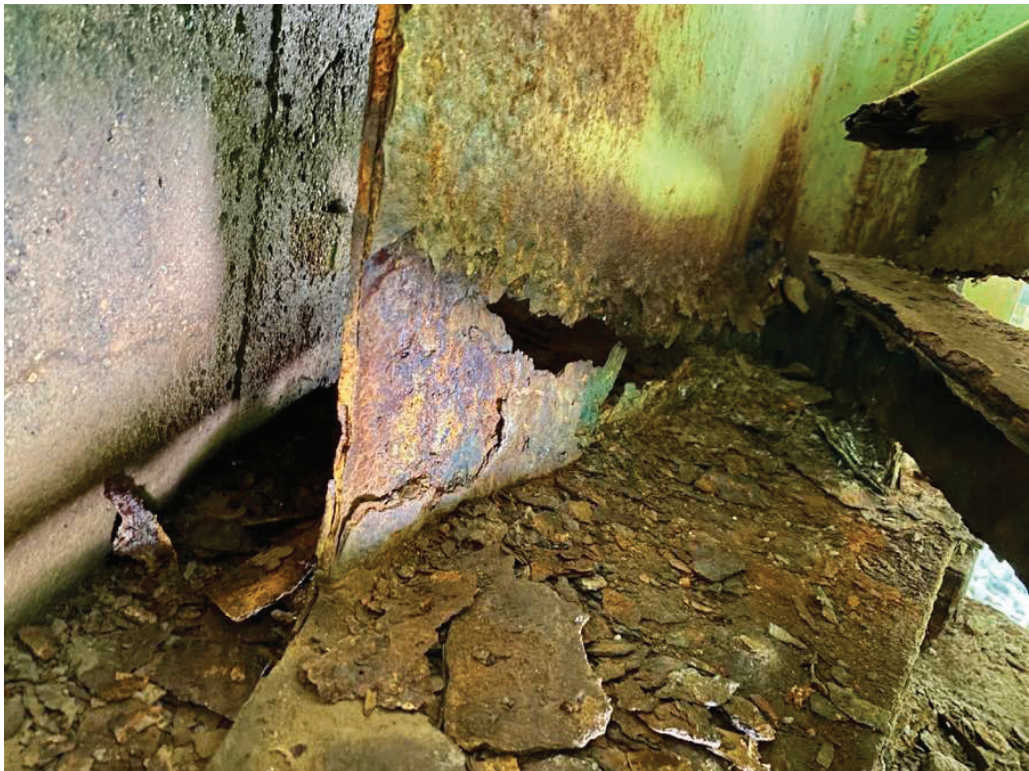
Photo 12: Girder 2 beyond the east bearing, with severe section loss and holes.
