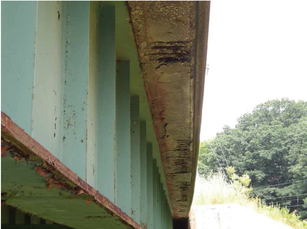
Photo 2: Underside of the North Deck Overhang in the West Span near midspan, looking west. Note the spalls.
