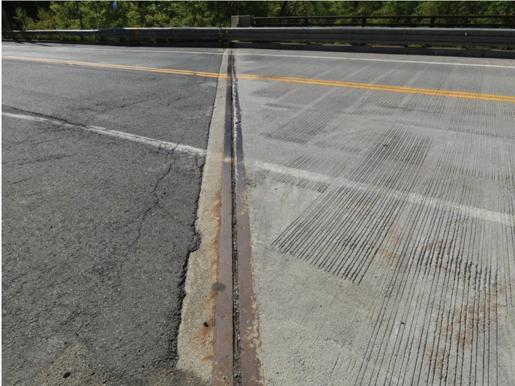
Photo 5: Gouges throughout the east abutment joint. Also, note the cracking in the adjacent approach pavement.
