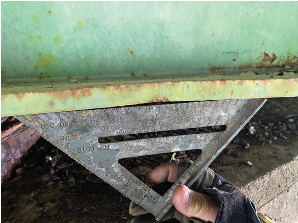
Photo 15: Girder 3 at east abutment, bottom flange bent upward.
