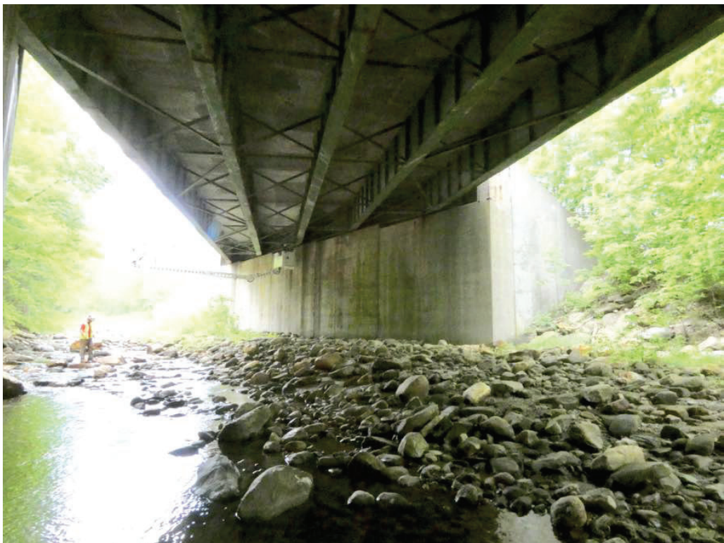
Photo 25: Aggradation in west half of channel, stream migrated to the east.
