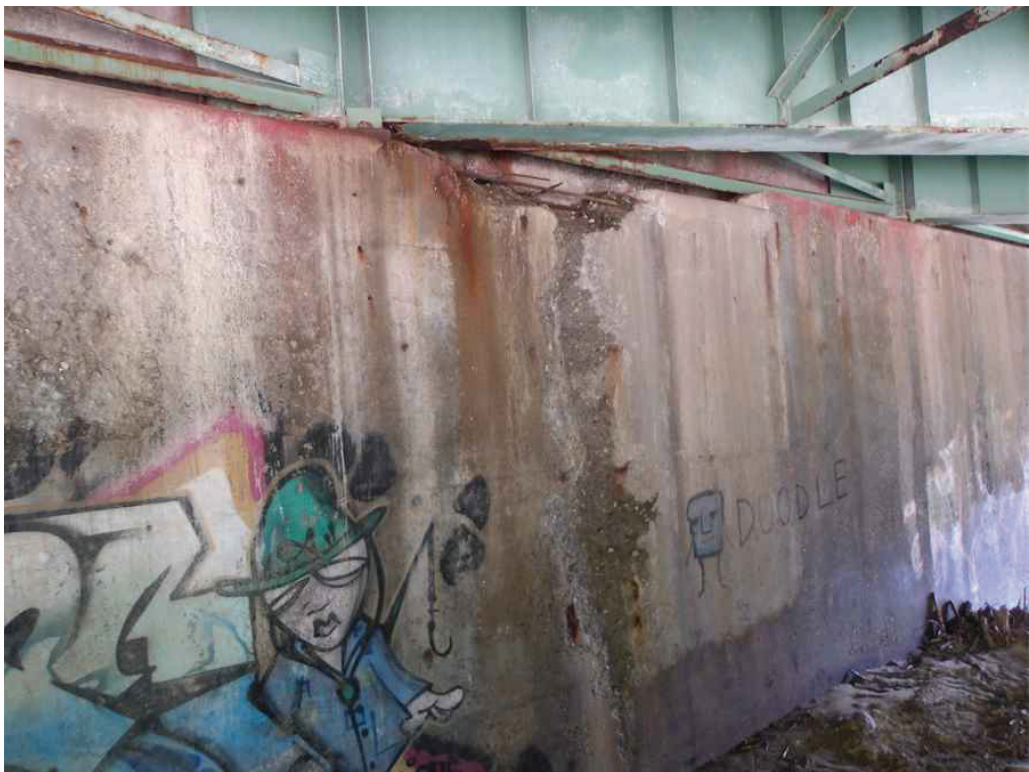
Photo 35: West Abutment below Bay 2, looking northwest. Note the spalls.
