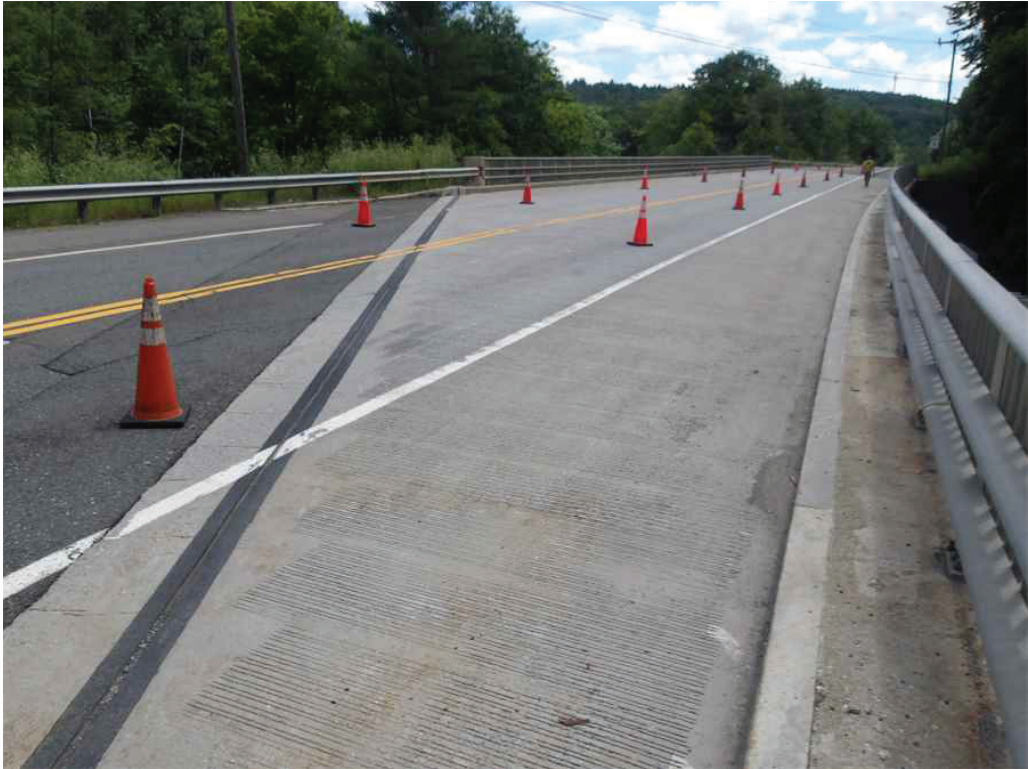
Photo 1: Top of the deck, looking northeast. Note the cracks.
