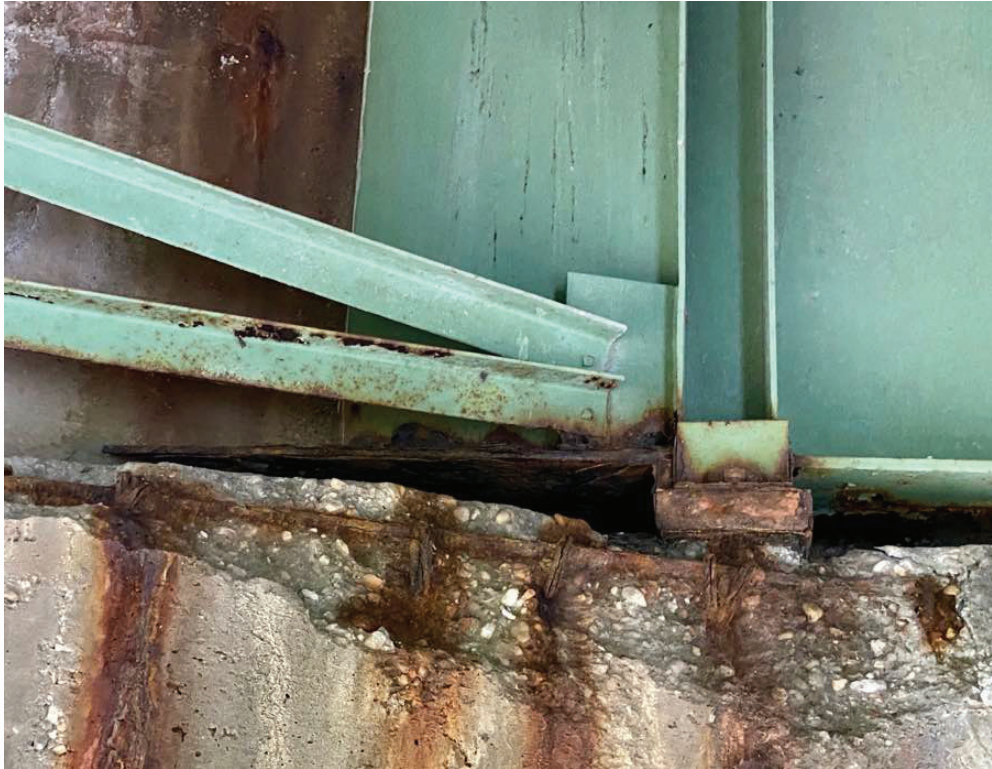
Photo 13: Girder 3 at west abutment, with heavy rust in bottom flange. Also note spall in bridge seat undermining the bearing.
