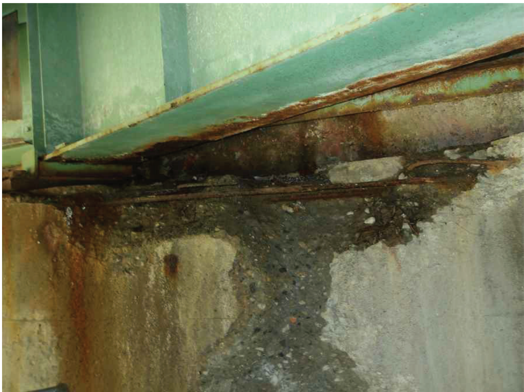
Photo 36: West Abutment below Bay 2 near Girder 3, looking west. Note the spall with exposed, debonded and broken rebar.
