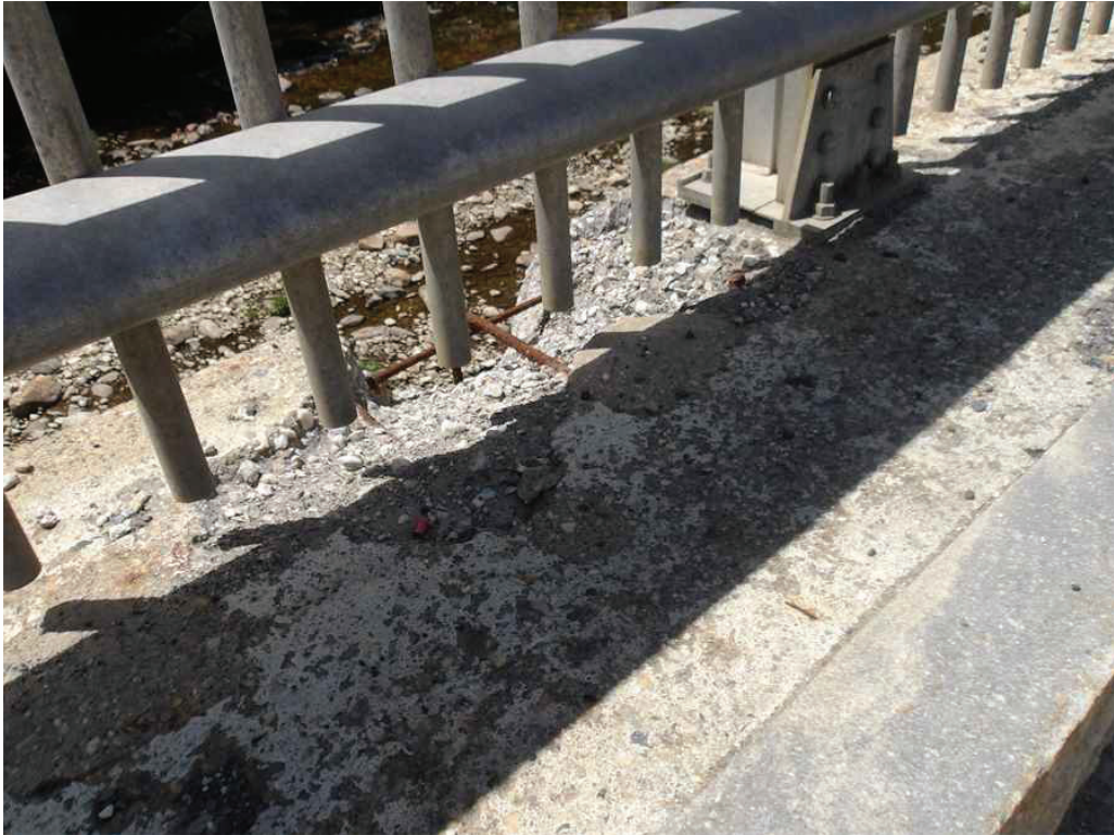
Photo 13: South Safetywalk in the West Span between the seventh and eighth post from the West Abutment, looking southwest. Note the spall and undermined post.
