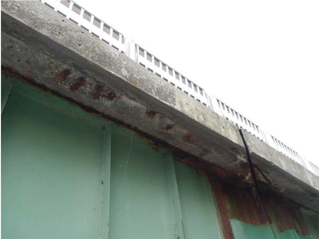
Photo 3: Underside of the North Deck Overhang at the Pier, looking southwest. Note the spalls.
