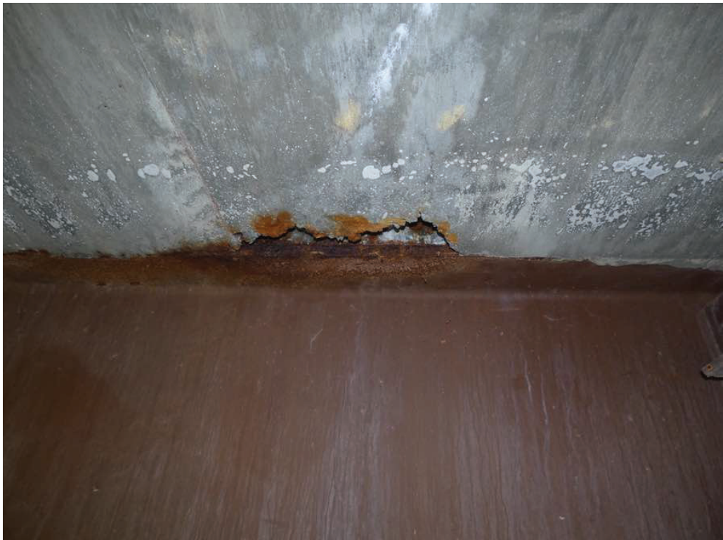
Photo 4: Spall and hollow area adjacent to beam 8, near the east end.
