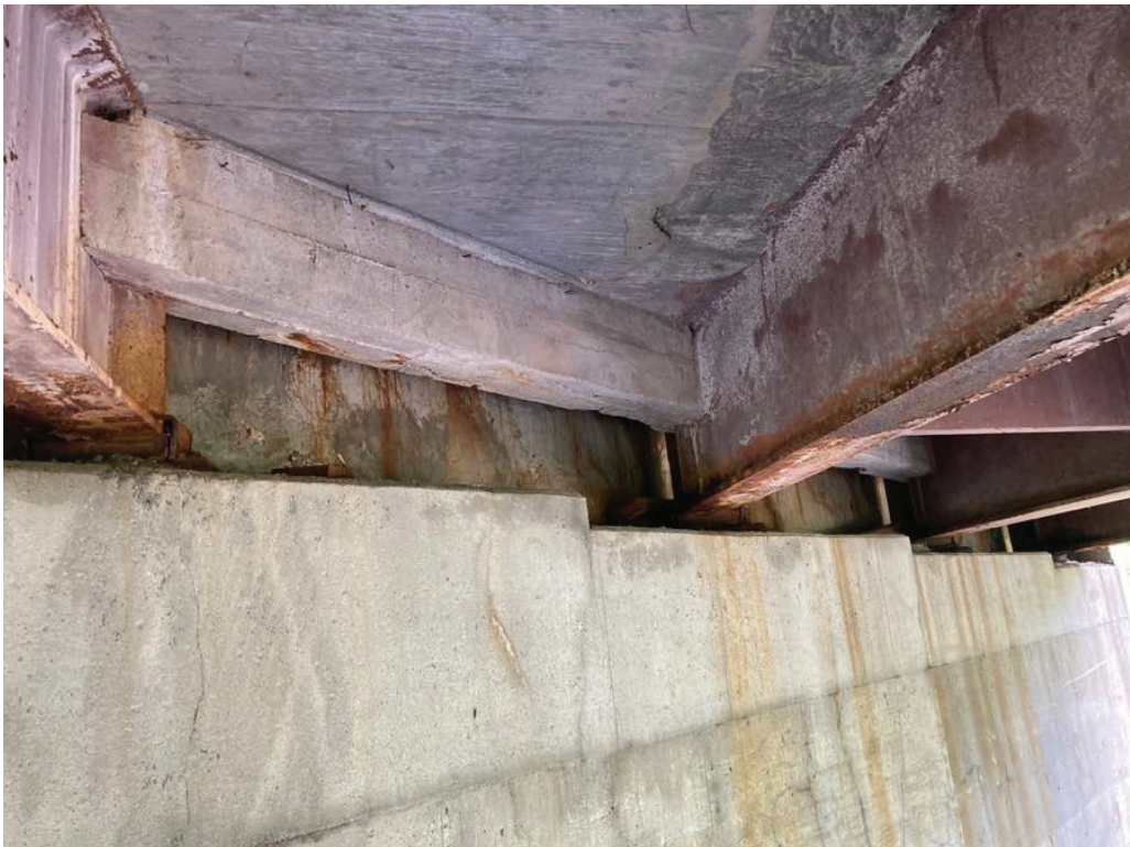
Photo 8: Typical cracking and spalling of the end diaphragms, bay 3 at the west abutment shown.
