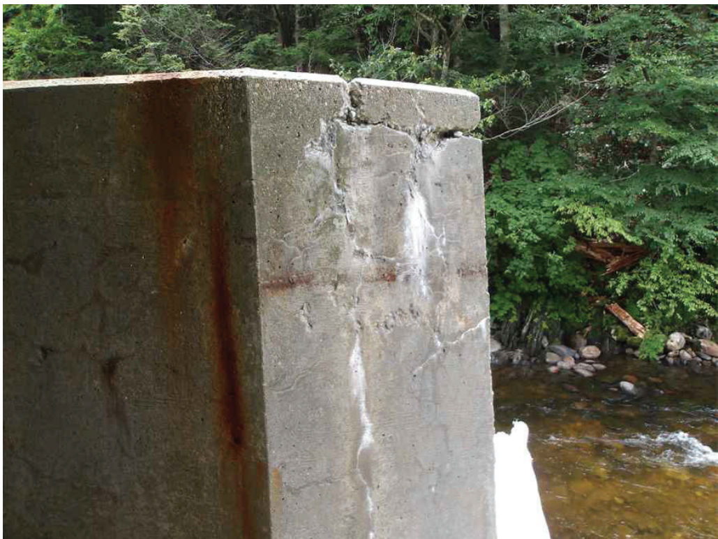
Photo 47: West side of the Pierwall at the south end, looking east. Note the spall and cracking.
