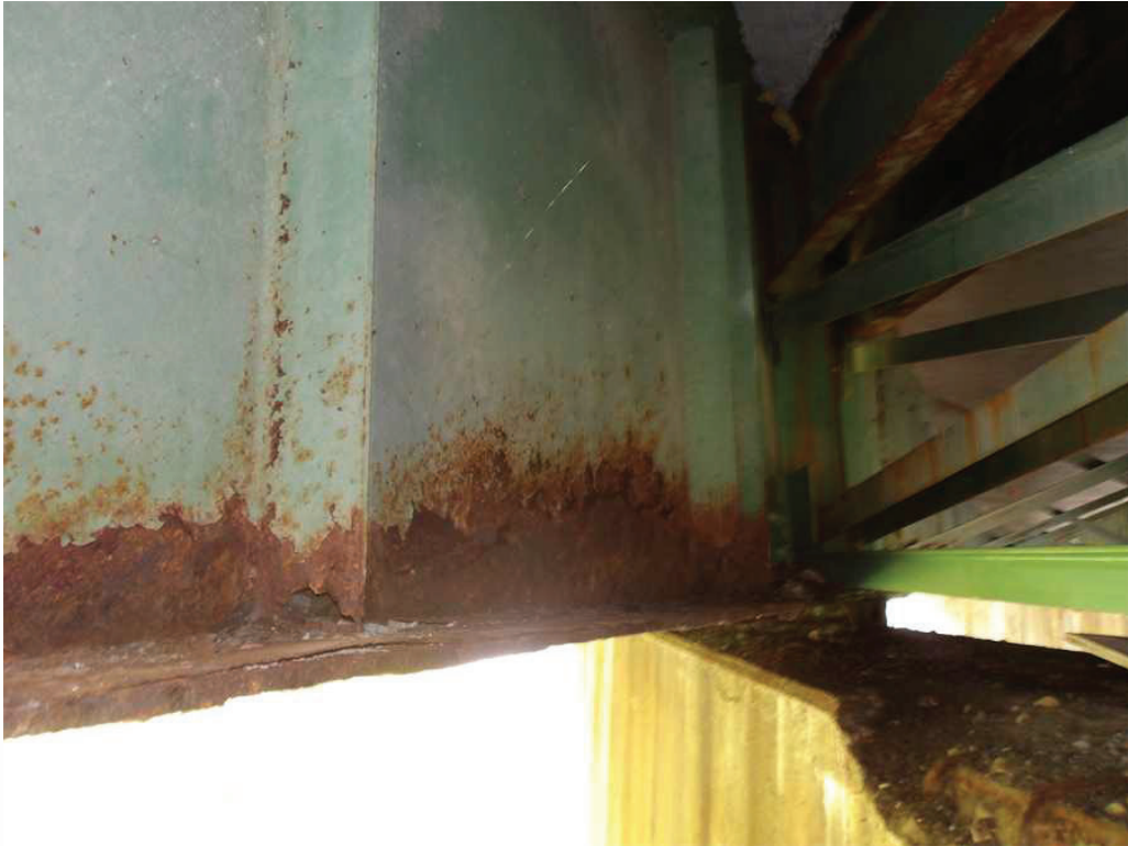
Photo 27: South side of Girder 3 at the Pier, looking northeast. Note the areas of section loss and the stiffener rust holes.
