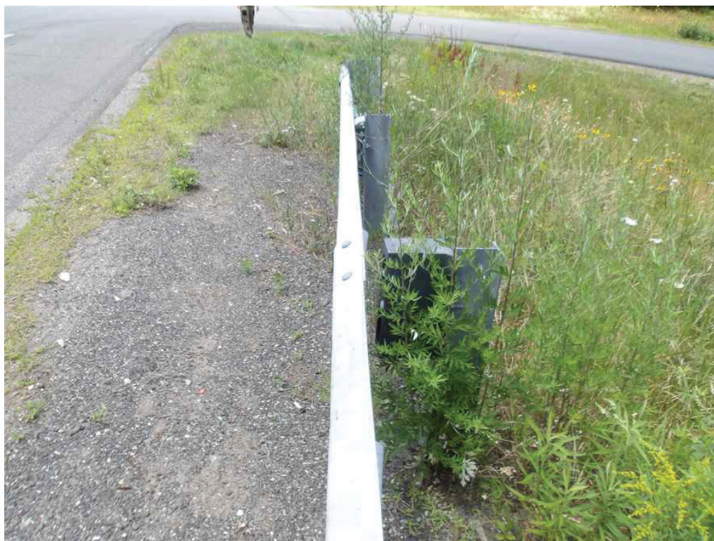
Photo 51: End of the northwest guardrail, looking west. Note the disconnected post and the loose/leaning end.
