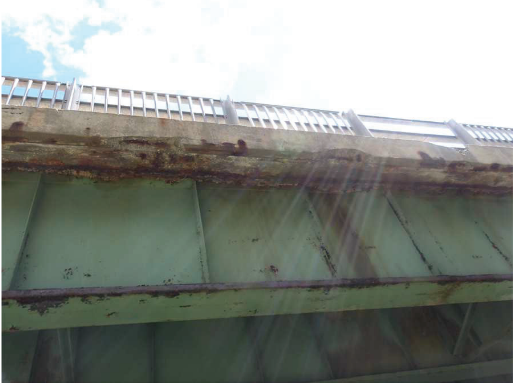
Photo 6: Underside of the South Deck Overhang in the West Span between the third and fourth intermediate cross frames from the West Abutment, looking north. Note the spalls on the deck and the safetywalk.
