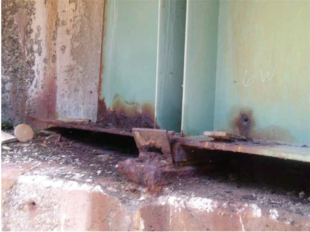
Photo 24: South side of Girder 6 and the bearing at the West Abutment, looking northwest. Note the bent bottom flange, section loss, drilled hole in the web, rusted bearing, and bent keeper plate with a rust hole.
