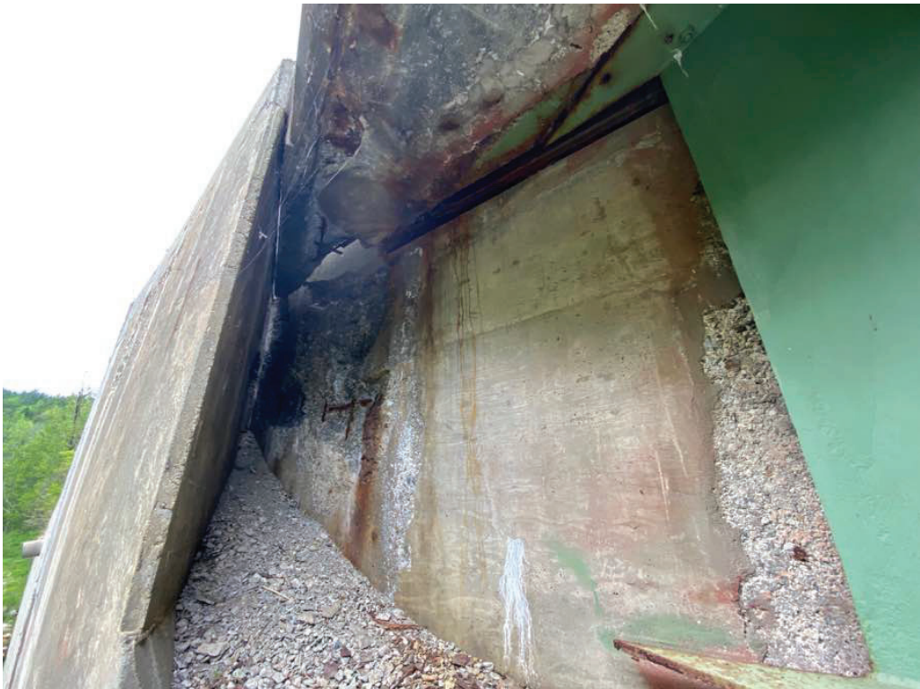
Photo 18: Southwest cheekwall and backwall, Note heavy scaling and spalling with exposed rebar, and heavy debris buildup on bridge seat.
