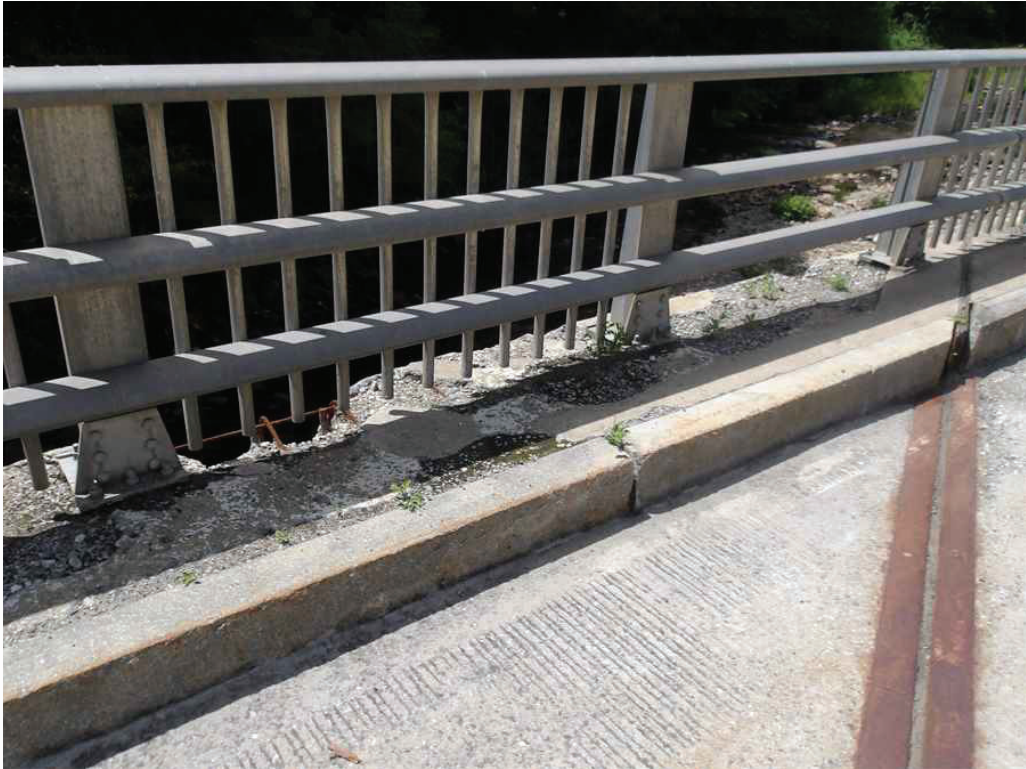
Photo 15: South Safetywalk in the East Span between the first and third post from the Pier, looking southwest. Note the spalls, undermined post, and missing pickets.
