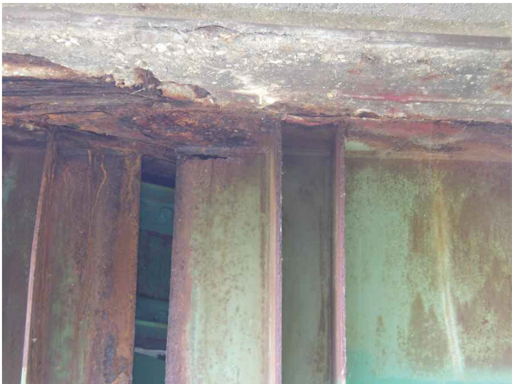
Photo 25: North side of Girder 1 at the Pier, looking south. Note the rust hole and deck joint steel plates in contact with the girder top flanges.
