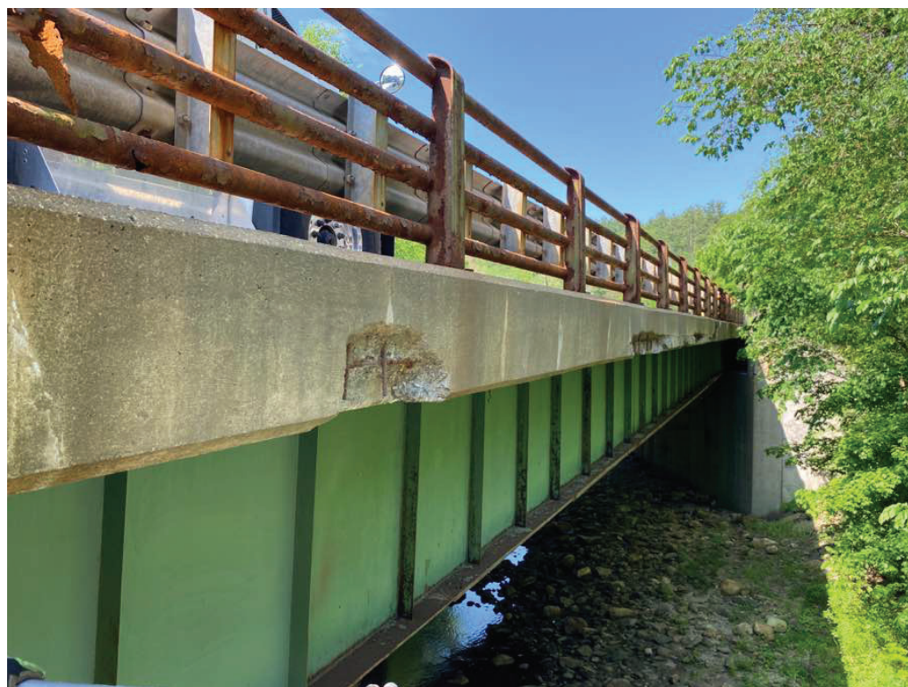
Photo 6: North deck fascia with several spalls.
