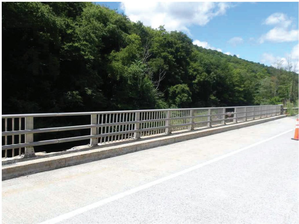
Photo 19: South Bridge Railing in the West Span, looking southwest. Note the missing pickets.
