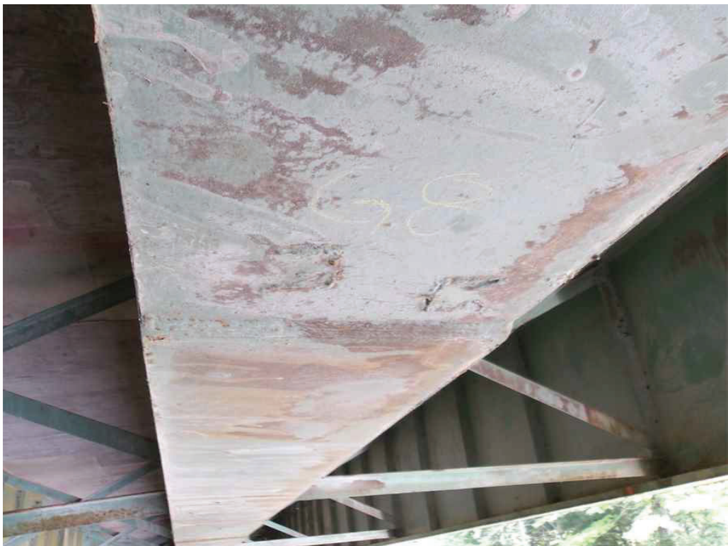
Photo 31: Underside of Girder 8 near the East Abutment, looking west. Note the welded initials.
