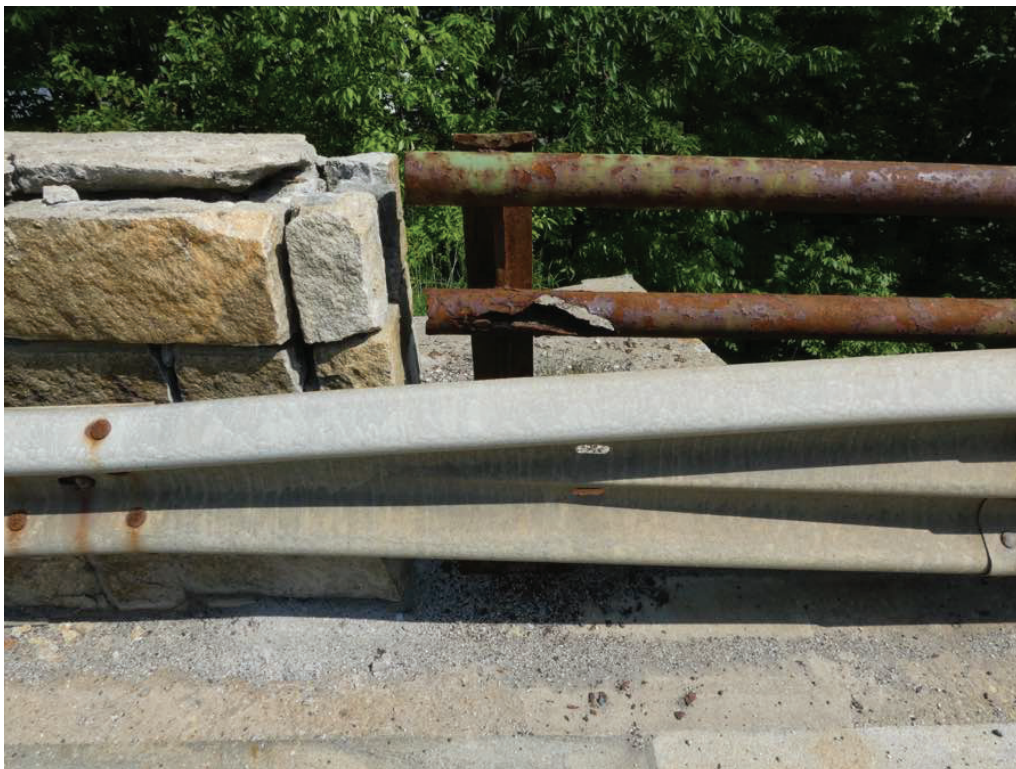
Photo 8: Northwest corner rail with corrosion holes in original bridge rails. Also note deteriorated cap and loose concrete blocks in end post.
