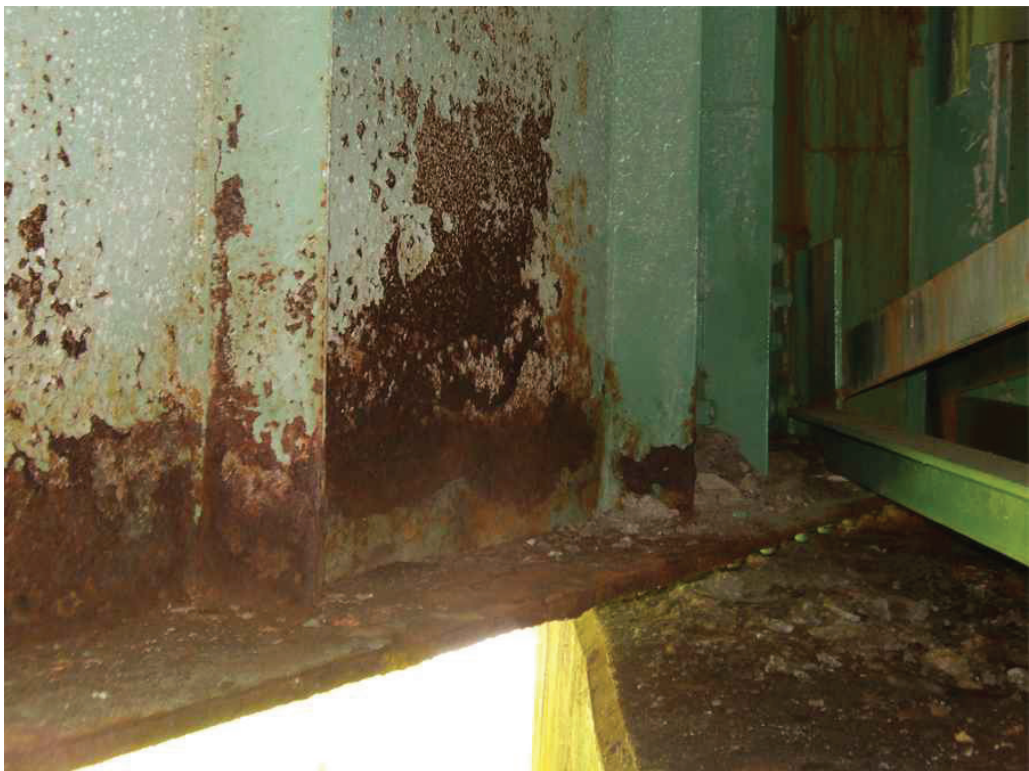
Photo 26: South side of Girder 2 at the Pier, looking northeast. Note the areas of section loss and the stiffener rust hole.
