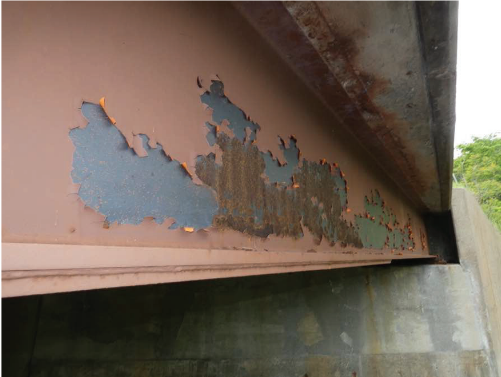
Photo 9: Area of missing paint on the south face of beam 14.
