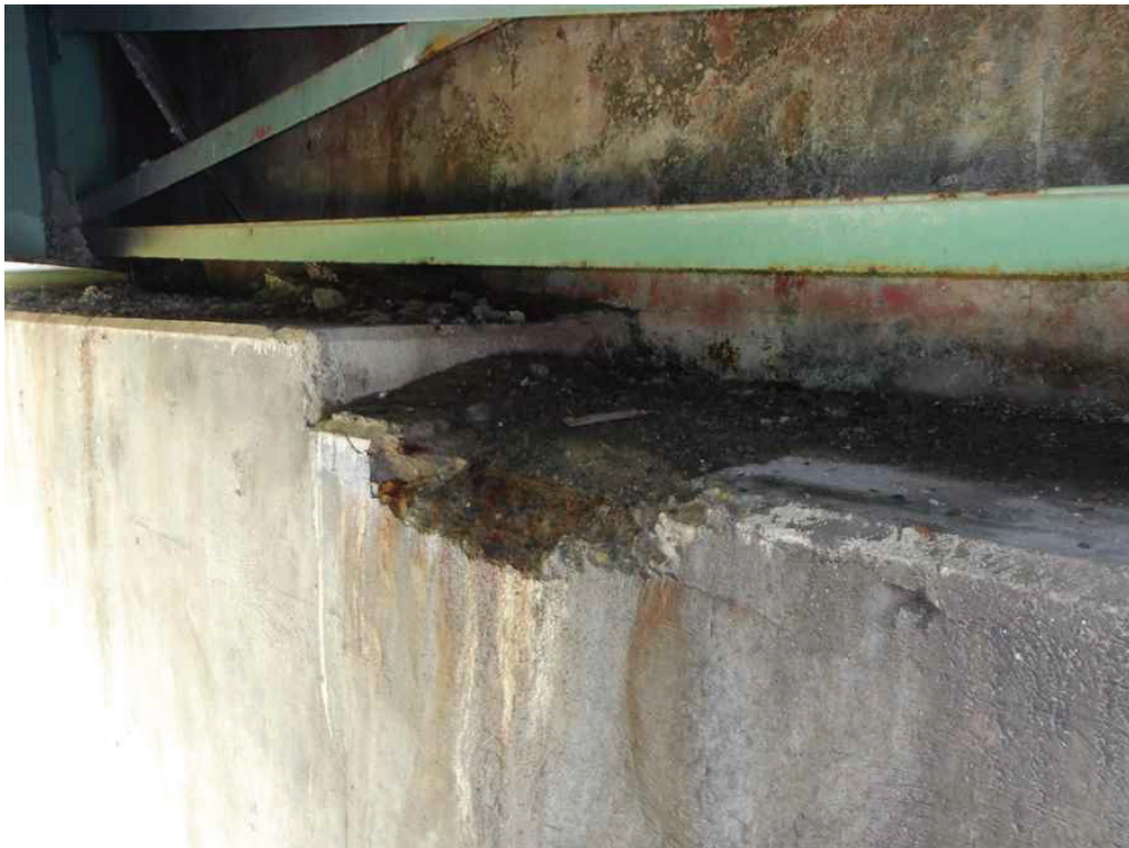
Photo 40: East Abutment below Bay 2, looking northeast. Note the spall.
