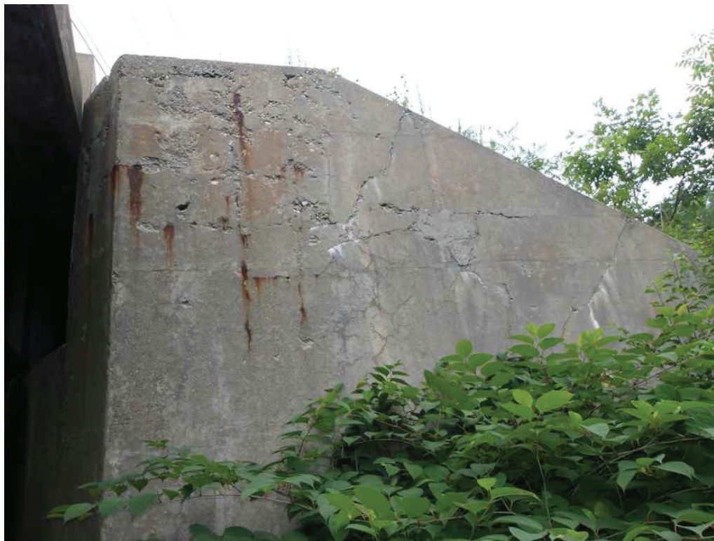
Photo 43: Northwest Wingwall, looking west. Note the scaling and cracking.
