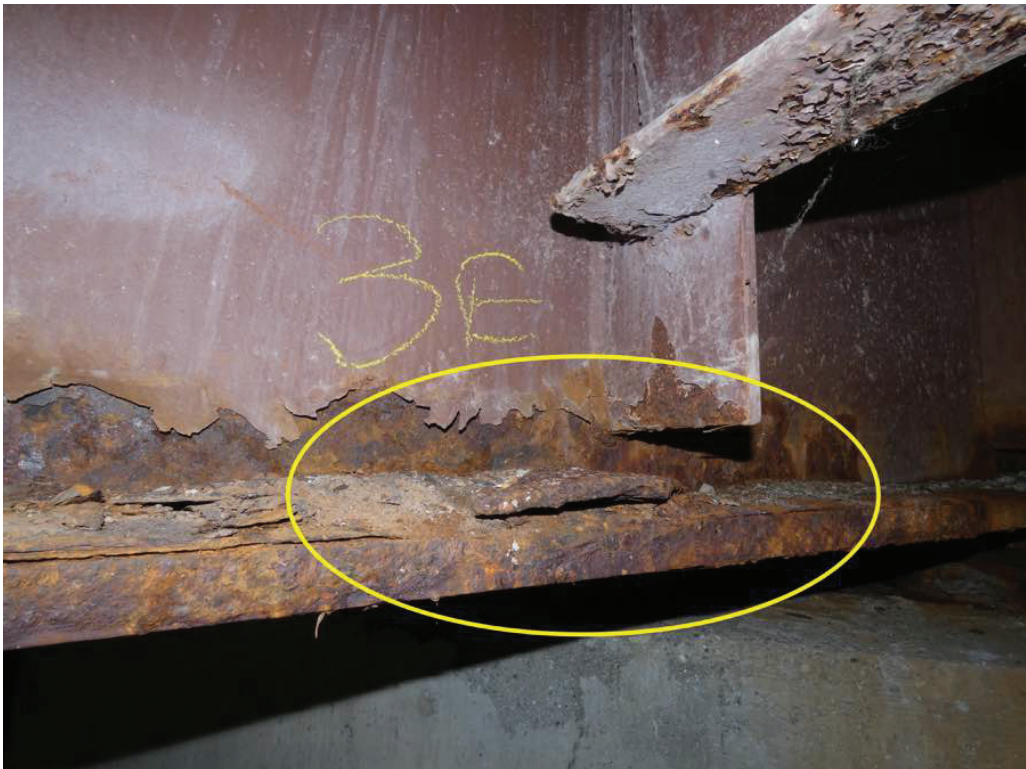
Photo 6: Plate welded to the top of the bottom flange near the east end of beam 3.
