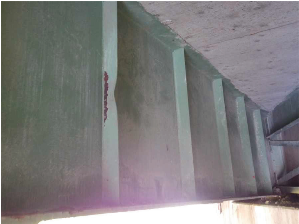
Photo 32: South side of Girder 11 near the East Abutment, looking northeast. Note the bent stiffener.
