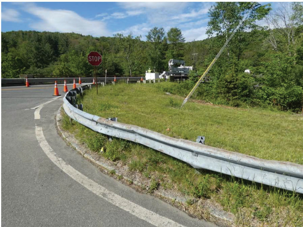
Photo 14: Minor damage to guardrail panels in the northeast approach guardrail.
