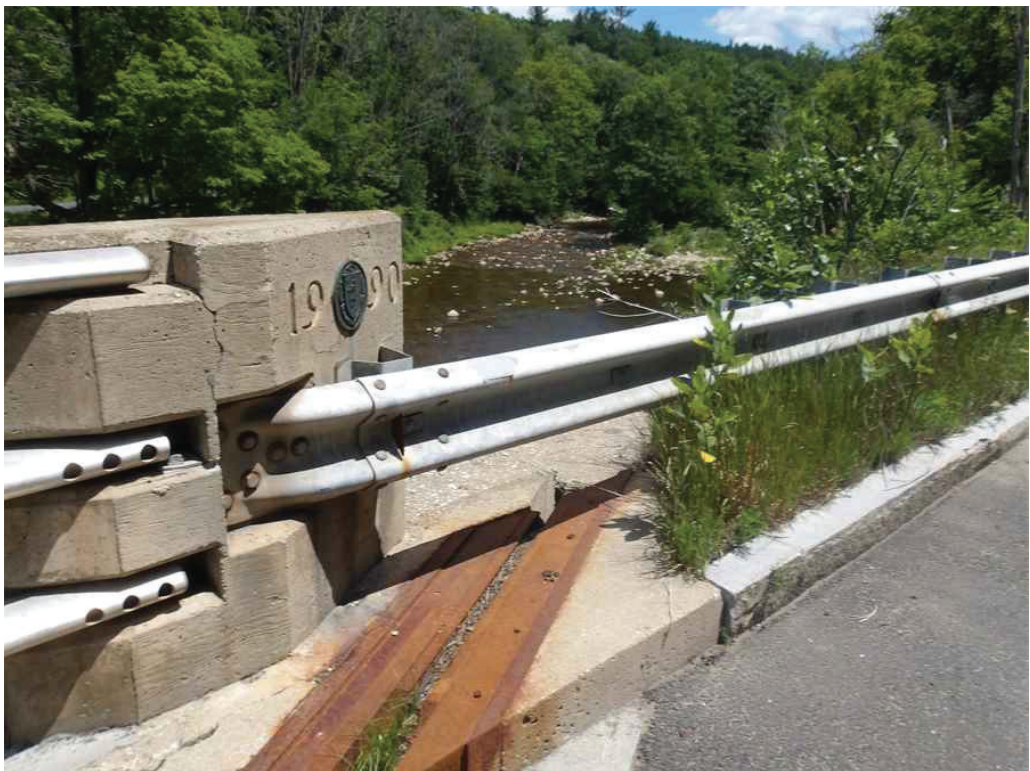
Photo 50: Northeast guardrail transition, looking north. Note the missing post.
