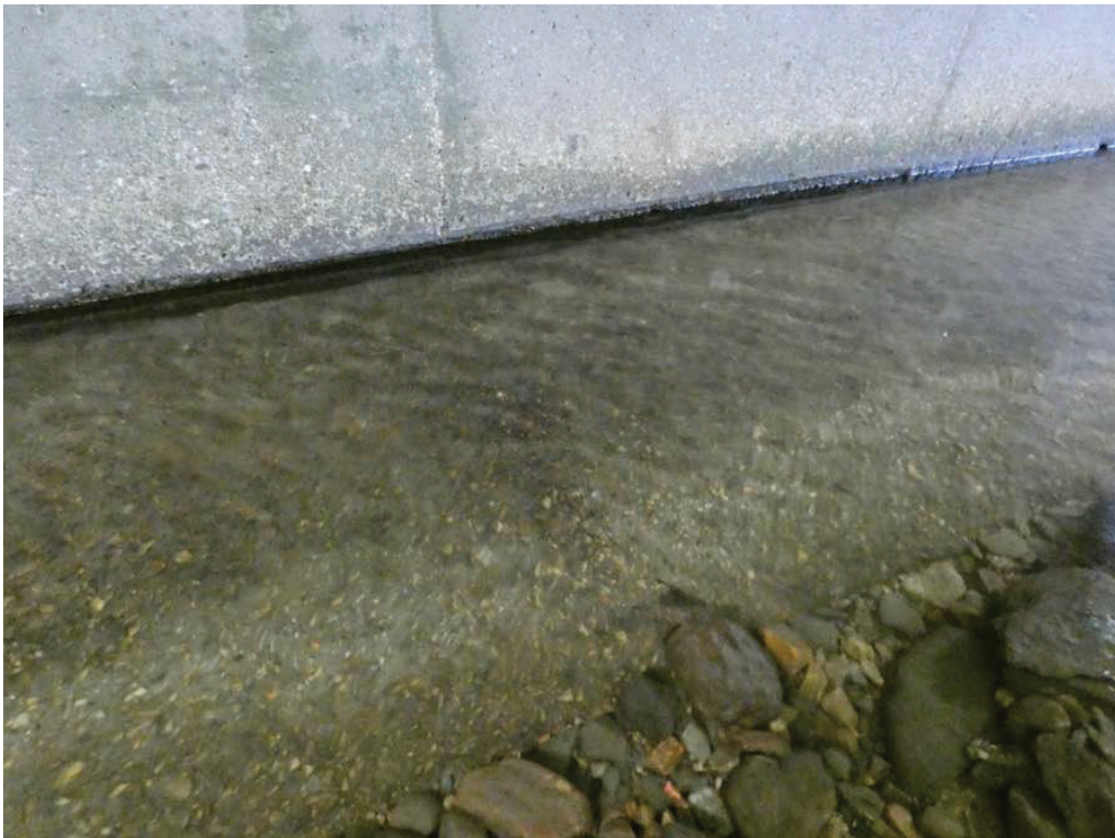
Photo 24: East abutment footing exposed and flush with streambed.
