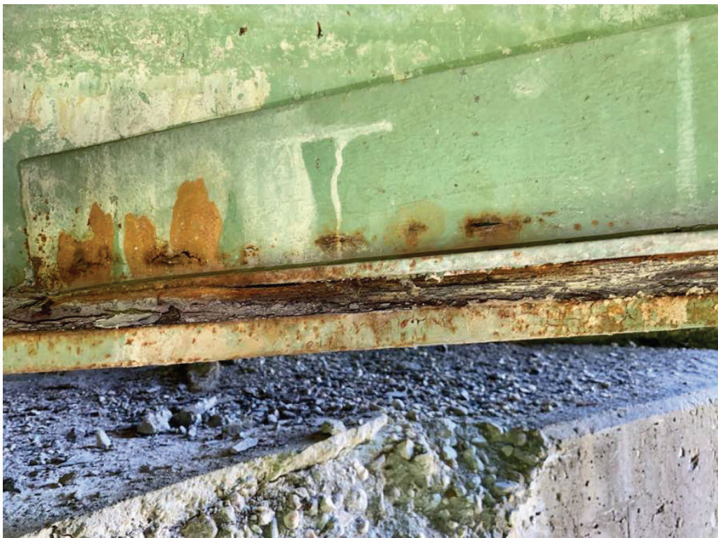
Photo 11: Girder 4 at west abutment, with pack rust between bottom lateral bracing and bottom flange (typical).
