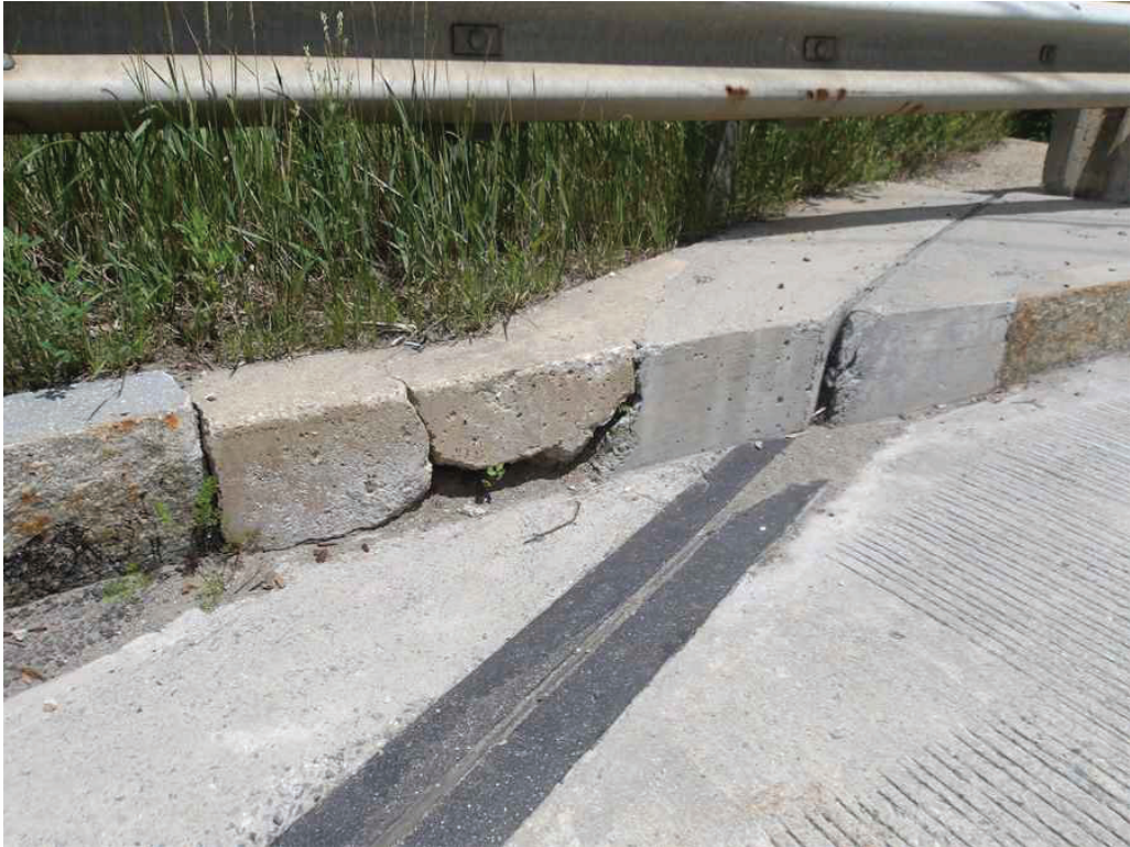
Photo 11: Northwest Approach Curb adjacent to the bridge, looking north. Note the crack and section of broken curb, and the safetywalk deck joint covered in concrete.
