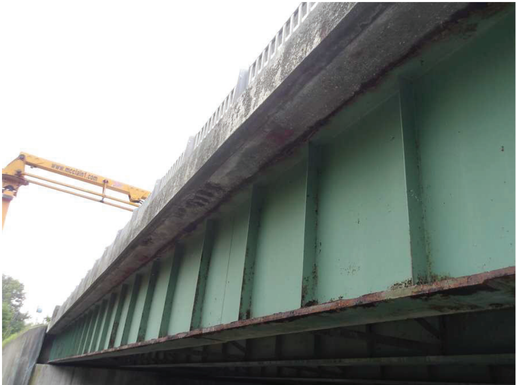
Photo 8: Underside of the North Deck Overhang in the East Span, looking southeast. Note the spalls.
