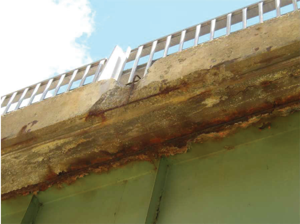
Photo 4: Underside of the South Deck Overhang in the West Span between the first and second intermediate cross frames from the West Abutment, looking north. Note the hollow areas, cracks, and the spall.
