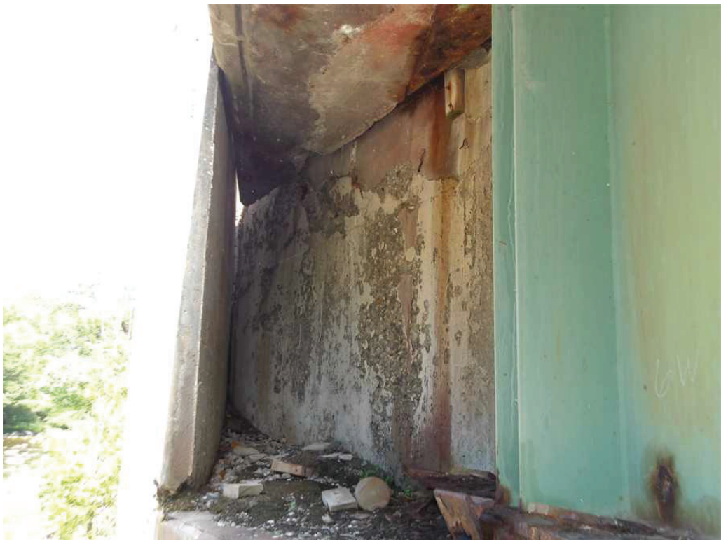
Photo 42: West Abutment backwall below the South Deck Overhang, looking southwest. Note the scaling.
