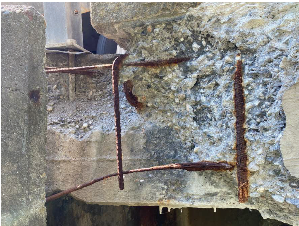
Photo 7: Northeast deck fascia spall with exposed rebar. Note undermining of masonry end post and guardrail post.
