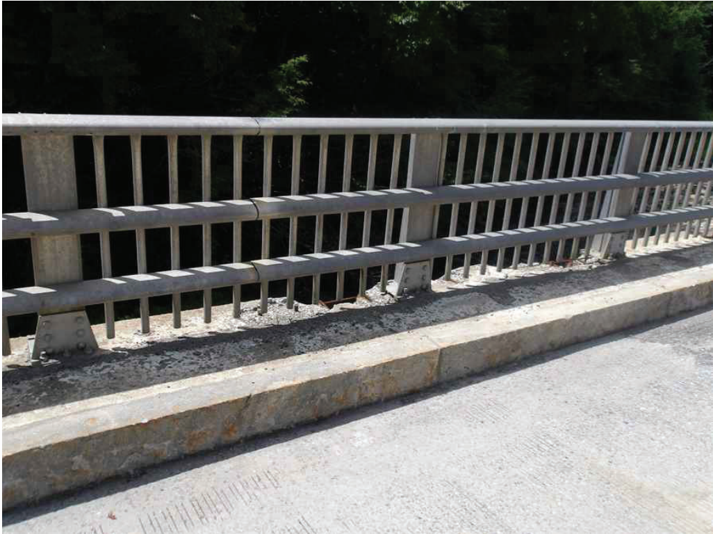
Photo 17: South Safetywalk in the East Span between the fifth and seventh post from the Pier, looking southwest. Note the spalls and undermined posts.
