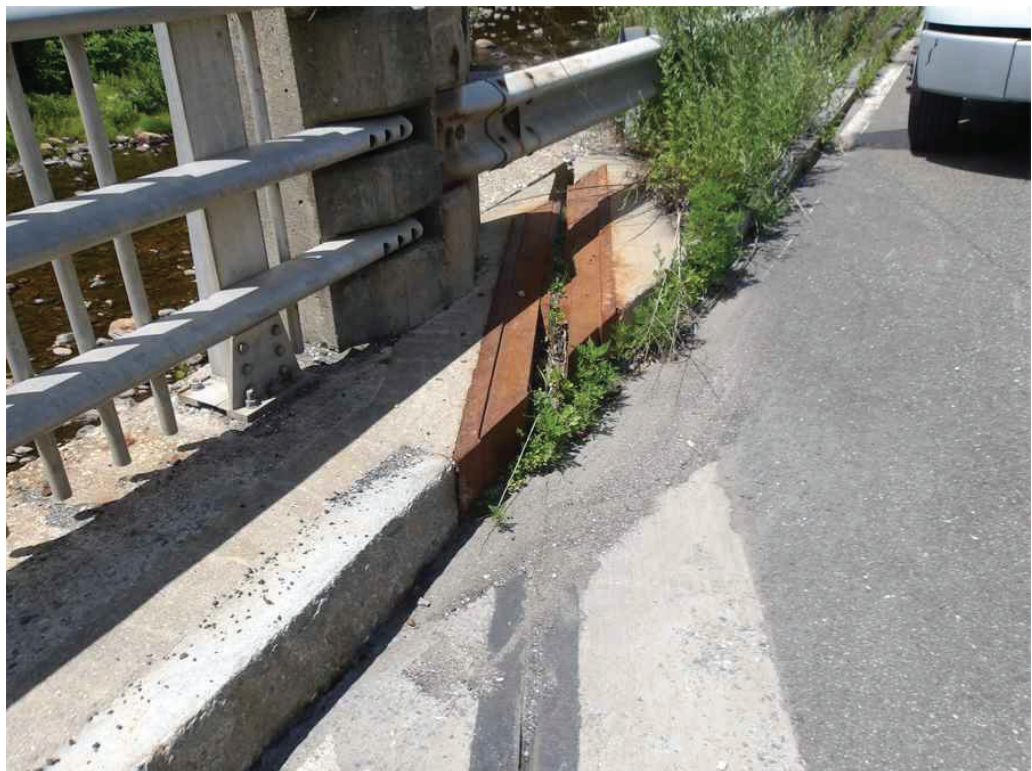
Photo 20: West Abutment Deck Joint in the South Safetywalk, looking southwest. Note the rust on the steel headers and the vegetation growth.
