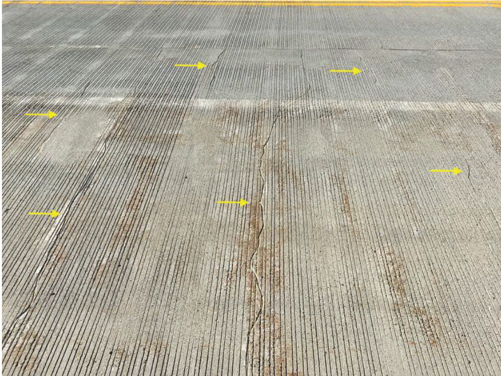
Photo 3: Wearing surface with transverse cracking. Typical.
