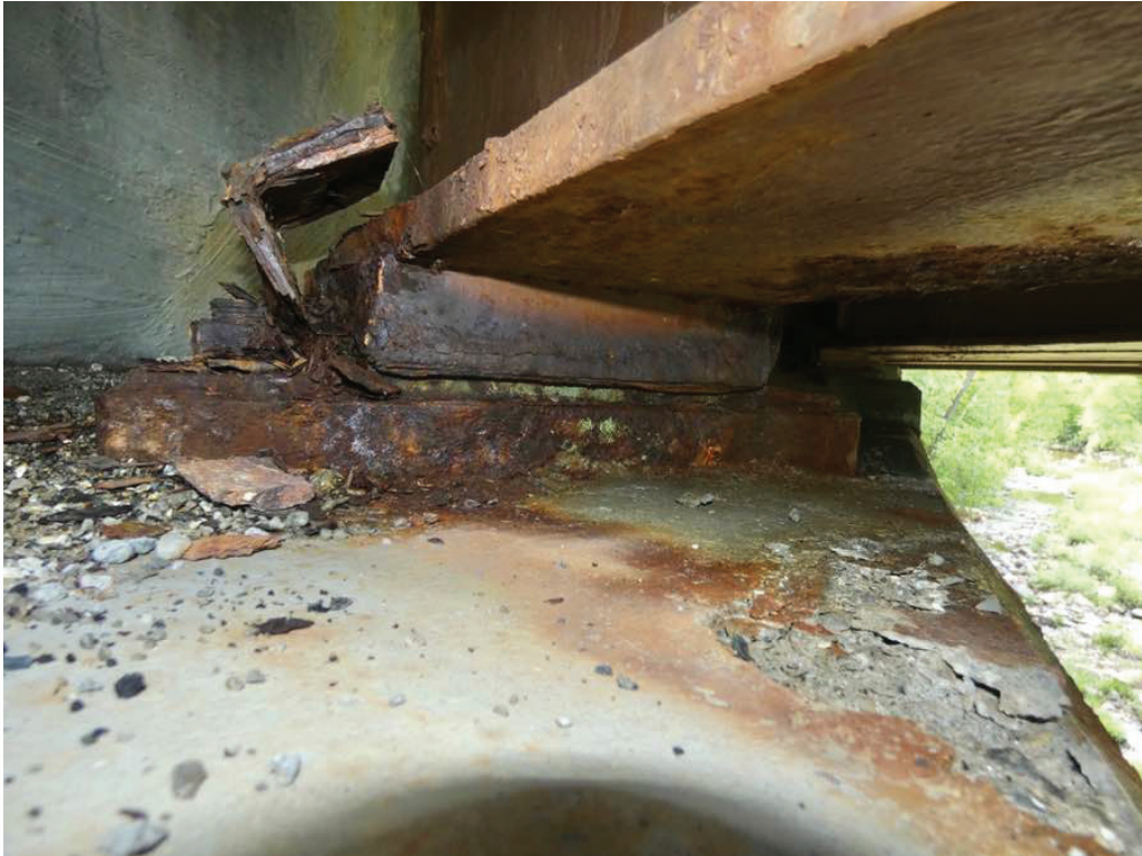
Photo 7: Bearing 8, east abutment, with pack rust and section loss to the keepers (typical).
