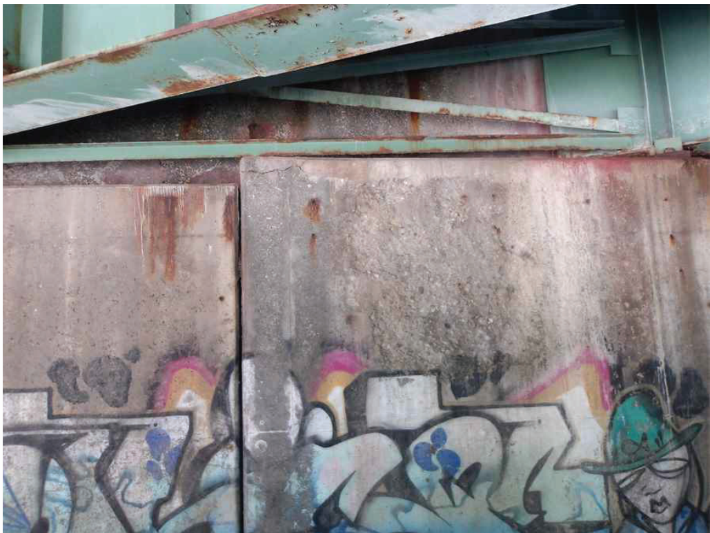
Photo 37: West Abutment below Bay 2, looking west. Note the crack, hollow area, and scaling.
