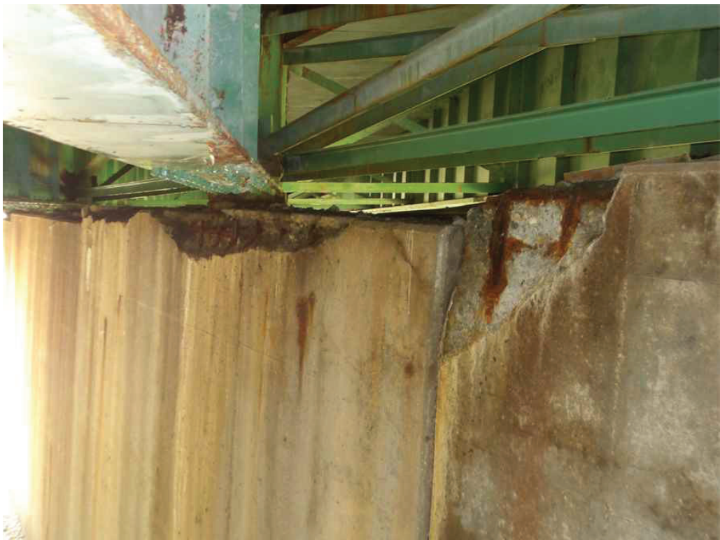
Photo 48: East side of the Pierwall below Bays 3 and 4, looking southwest. Note the spalls.
