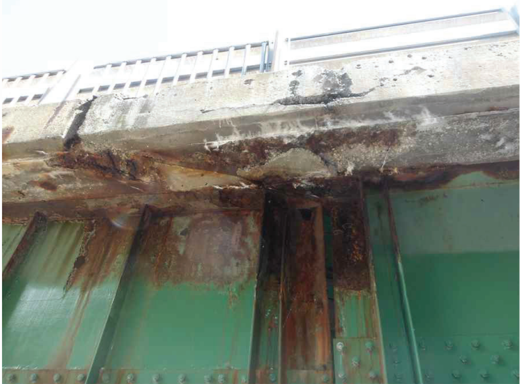
Photo 7: Underside of the South Deck Overhang at the Pier, looking north. Note the spalls on the deck underside and the vertical face of the safetywalk, and the rust holes on Girders 6 and 12.
