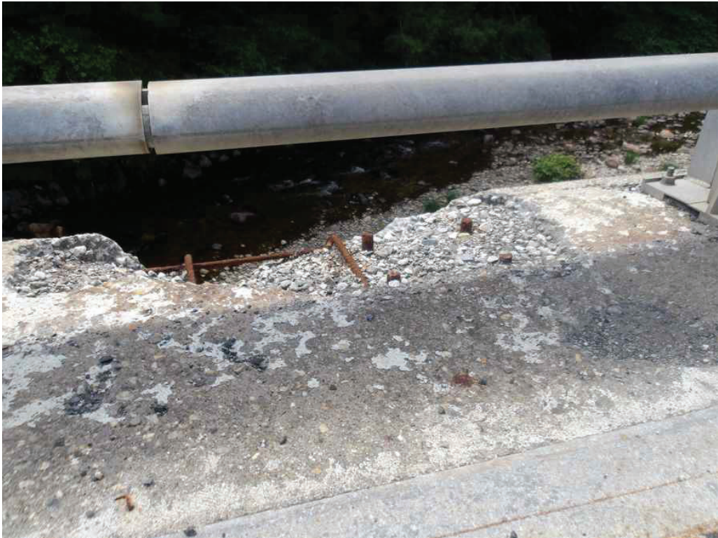
Photo 14: South Safetywalk in the West Span between the fourteenth and fifteenth post from the West Abutment, looking south. Note the spall.
