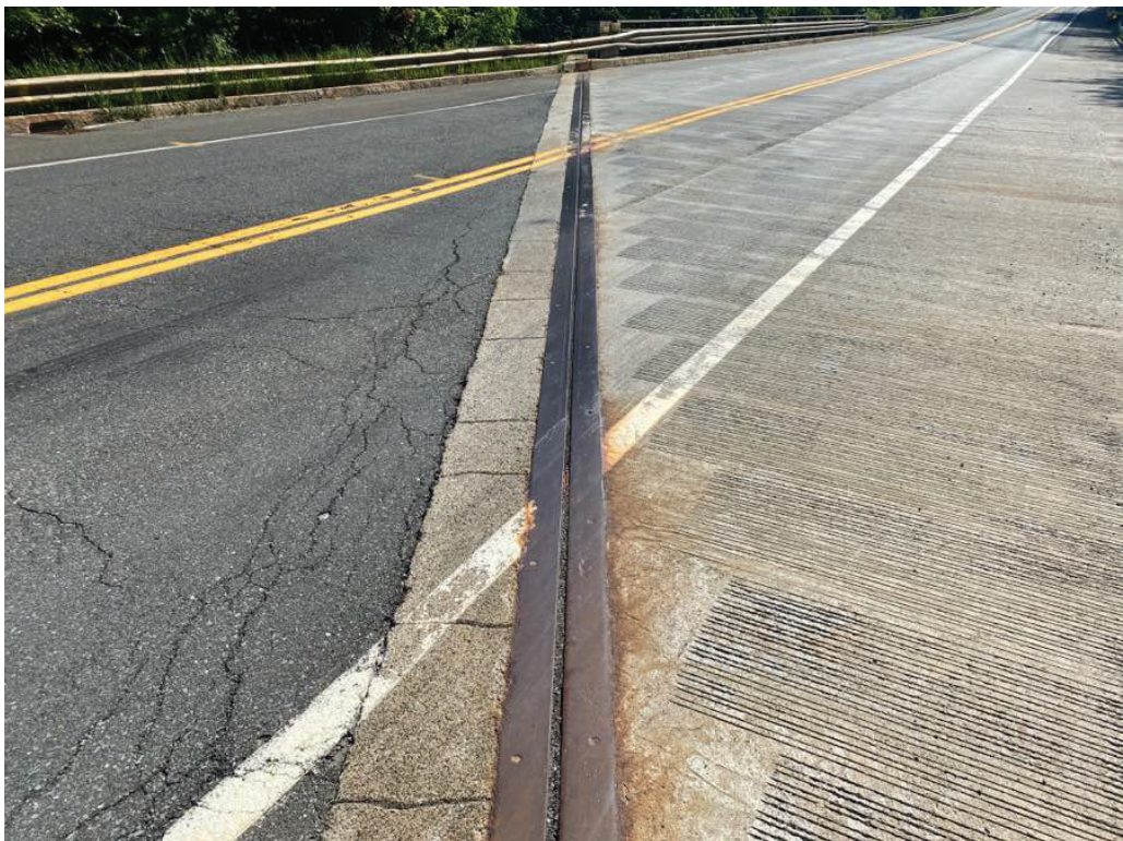
Photo 10: West deck joint with surface rust and debris. Note cracking in concrete joint header and in the approaches.
