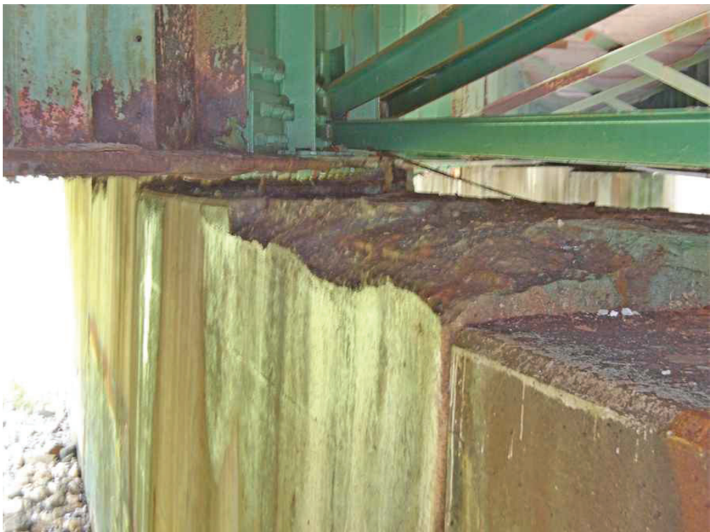
Photo 46: West side of the Pierwall below Bay 5, looking northeast. Note the spall.
