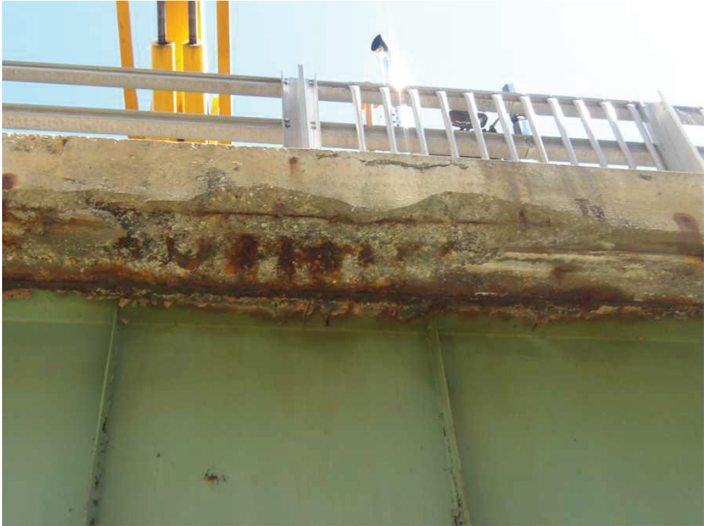
Photo 5: Underside of the South Deck Overhang in the West Span at the second intermediate cross frame from the West Abutment, looking north. Note the spalls on the deck underside and the safetywalk.
