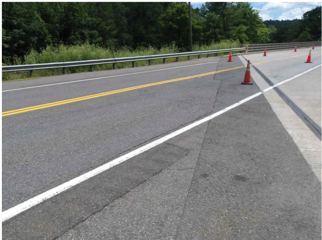
Photo 22: West Approach Pavement, looking northeast. Note the cracks.
