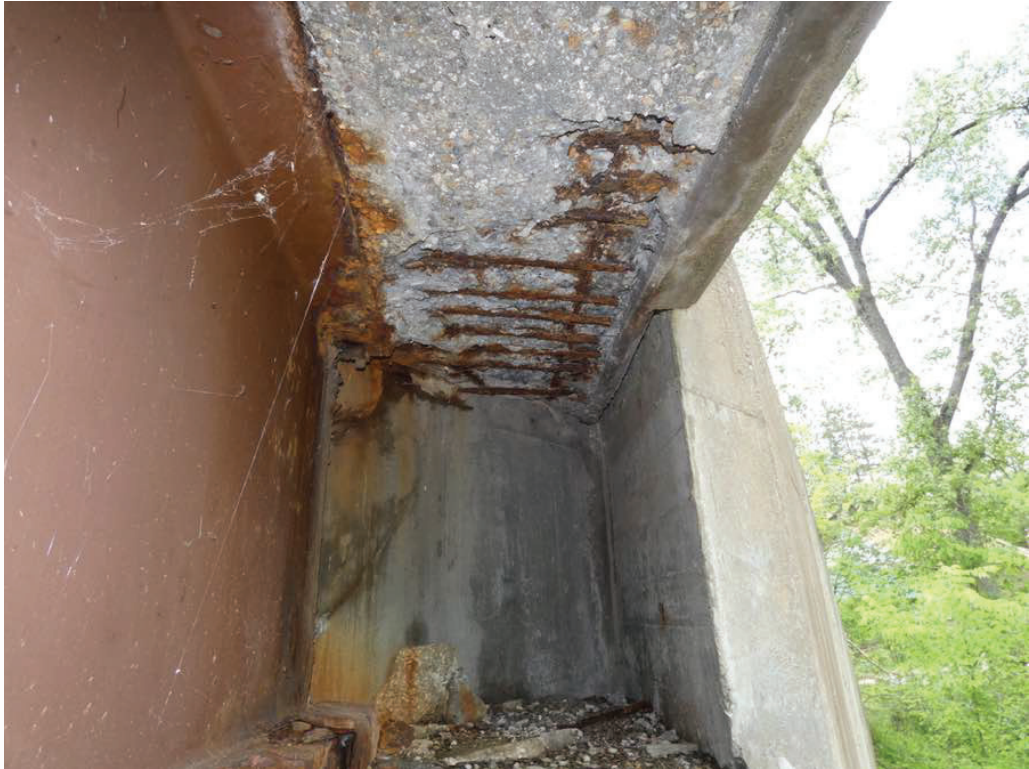
Photo 3: Spalling at the west end of the north overhang at the west abutment.
