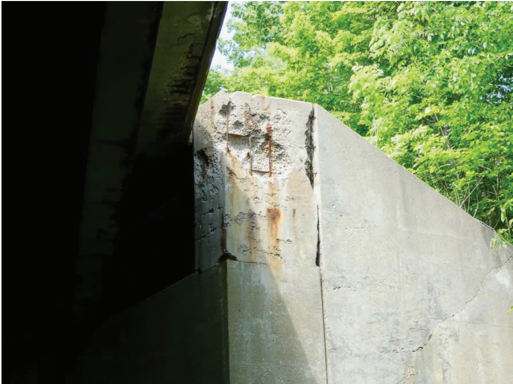
Photo 22: Northwest cheekwall, with spalls. Note diagonal crack in wingwall.
