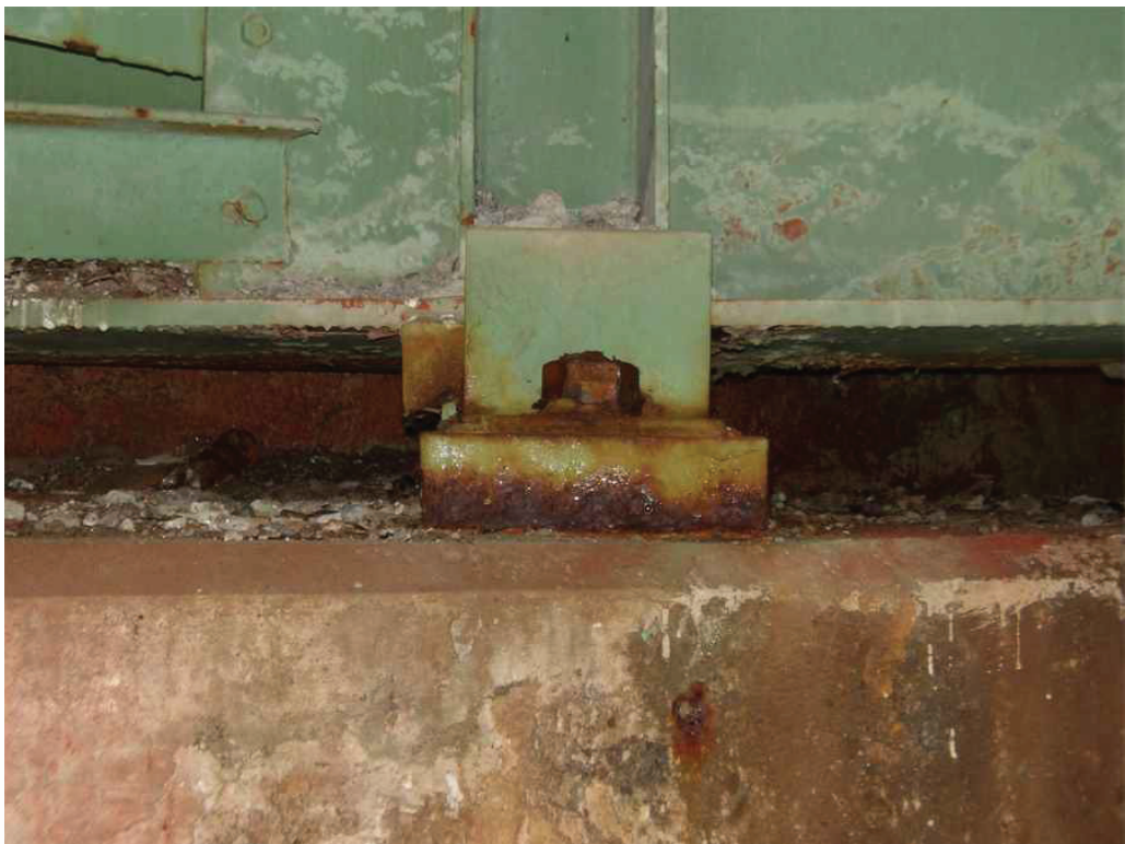
Photo 33: Girder 2 bearing at the West Abutment, looking west. Note the overhanging sliding plate.
