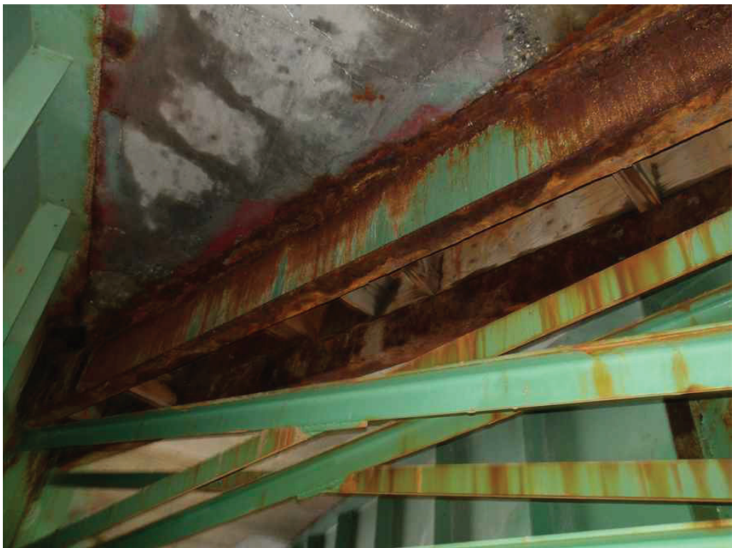
Photo 34: End cross frames at the Pier in Bay 4, looking northeast. Note the areas of heavy and laminated rust and the formwork.
