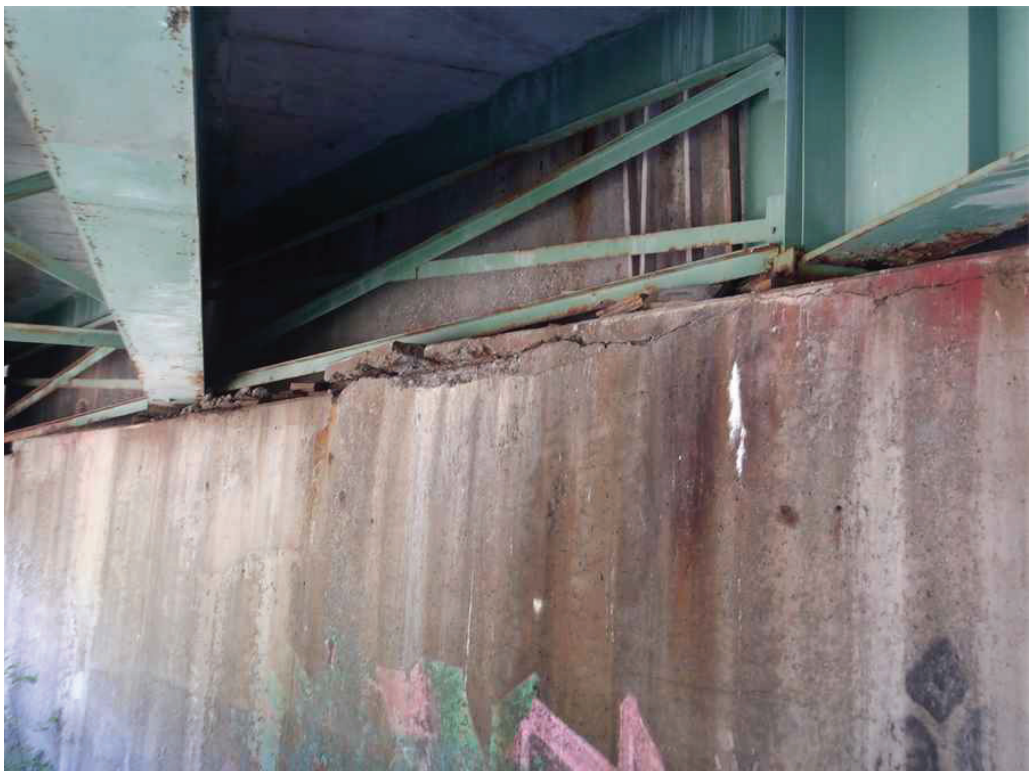
Photo 38: West Abutment below Bay 4, looking northwest. Note the spalls, exposed and debonded rebar, hollow area, and crack.
