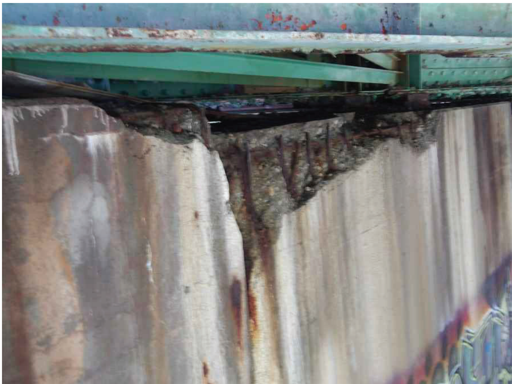
Photo 45: West side of the Pierwall below Bay 3, looking southeast. Note the spall.
