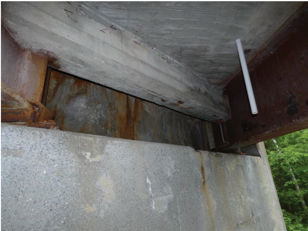
Photo 10: Spalling in the east backwall, bay 6.
