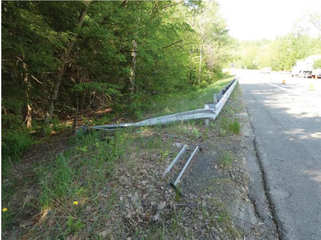
Photo 27: Collision damage at southeast guardrail end.
