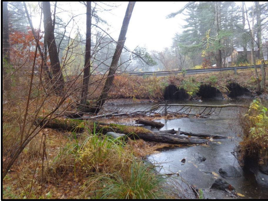
Photograph 5: View downstream showing the outfall structures on the upstream side of the bridge.
