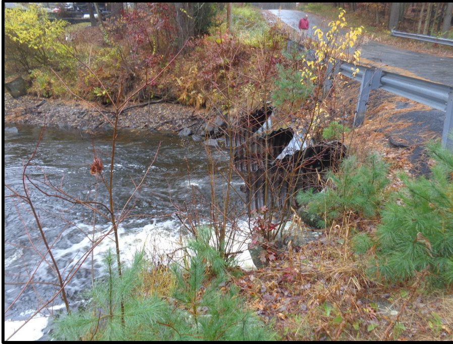
Photograph 9: View northwest of the outfall structures on the downstream side of the bridge.
