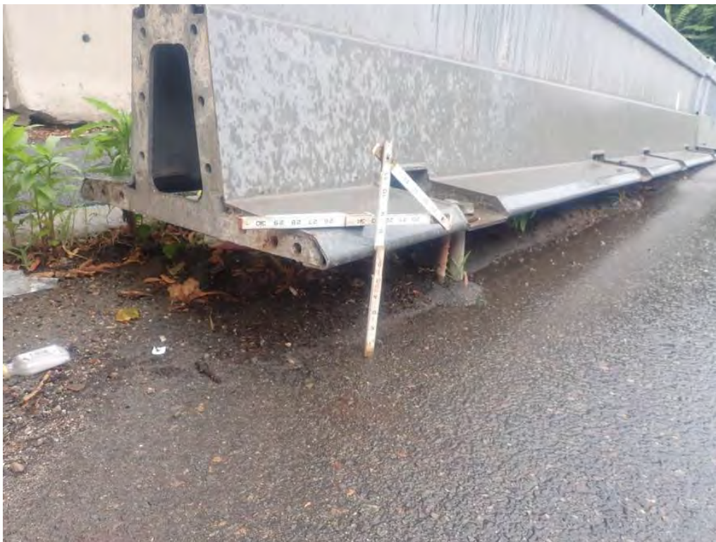
Photo 5: The last section of metal jersey barrier on the south end of the west railing has pulled up off the roadway with a 6" gap and can be moved by hand
