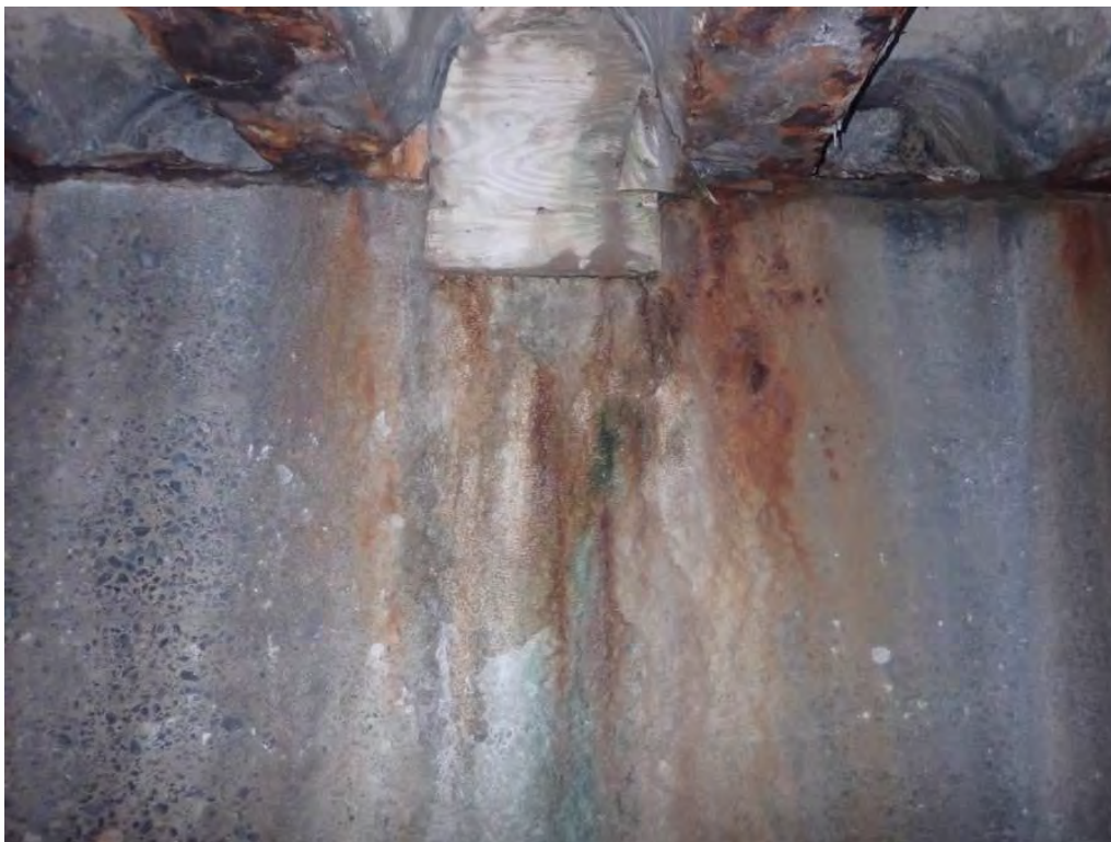
Photo 21: North breastwall, between beams #17 and #18, top half heavy efflorescence and rust staining with plywood form left at the top
