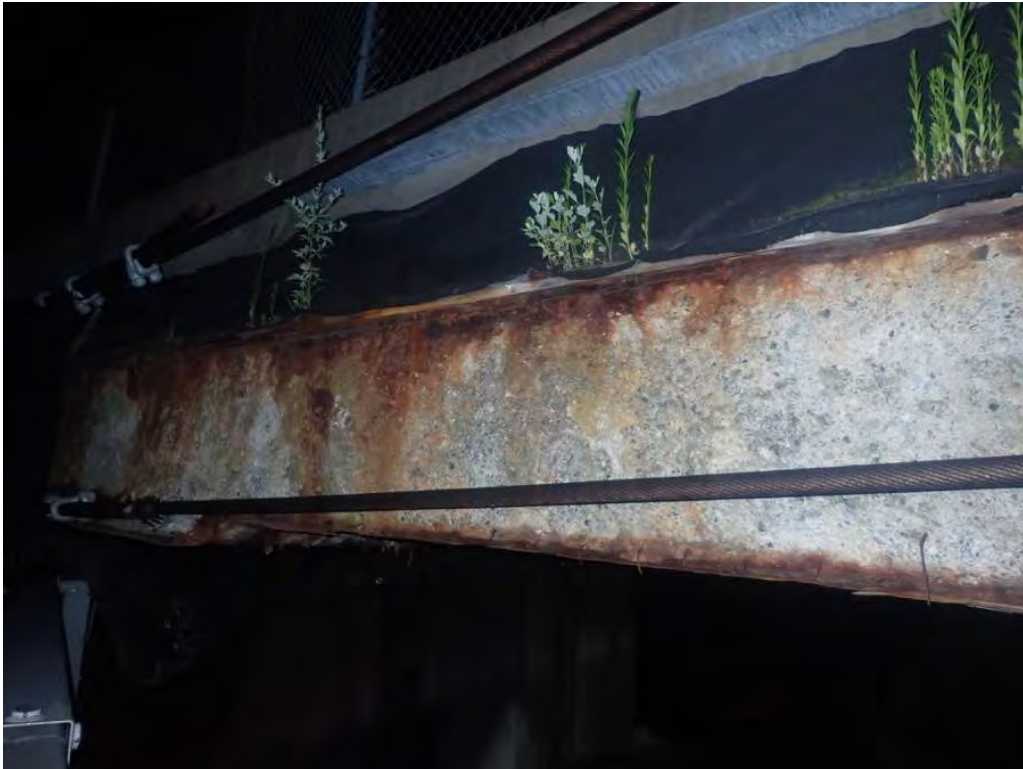
Photo 12: Beam #21, east fascia beam, with heavy spalling/ scaling concrete entire length with top and bottom flanges exposed
