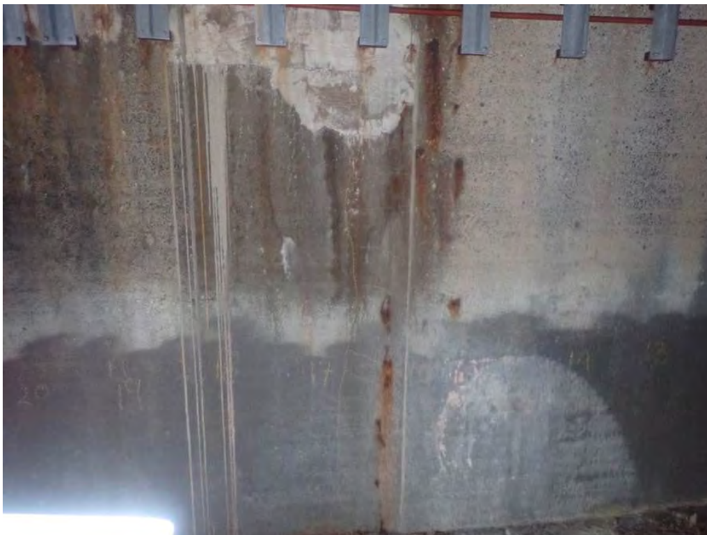
Photo 16: South breastwall, between beams #16 and #17, hollow concrete and hairline vertical crack with rust staining
