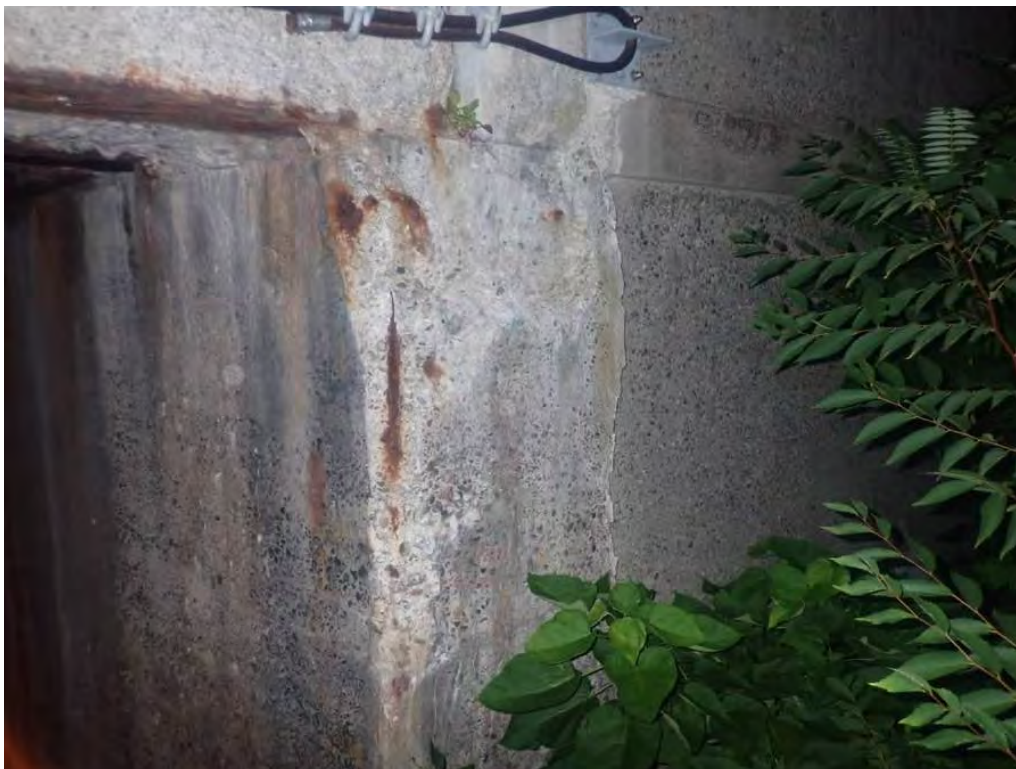
Photo 22: North breastwall, east end, is spalled with heavy scaling concrete, 5'-3" W x 7'-6" H x 10" D. Section loss to the exposed reinforcing at this location
