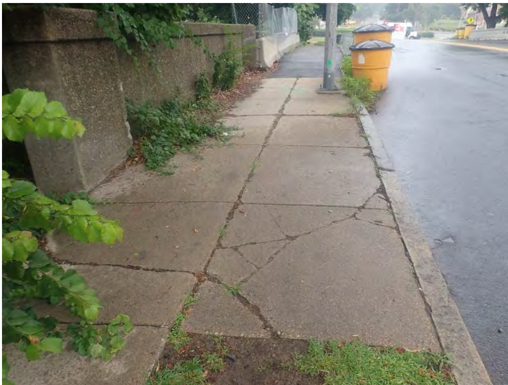
Photo 6: Southwest approach sidewalk, moderate cracking with minor spalling and vegetation between the panels
