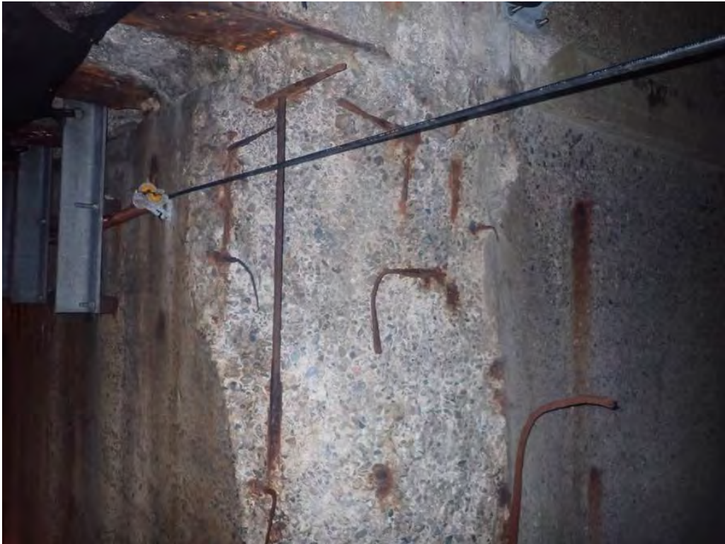
Photo 14: South breastwall west end, close up at the top
