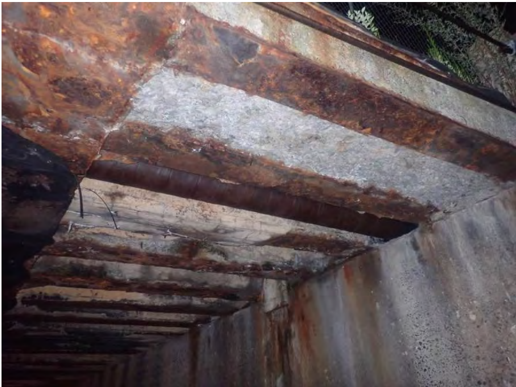
Photo 8: Beams #15 through #21, typical heavy rusting to exposed bottom flange
