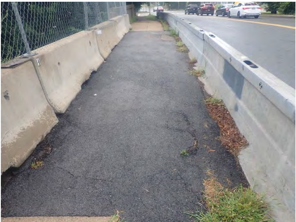
Photo 4: Original concrete parapet removed and replaced with concrete jersey barrier and chainlink fence as pedestrian railing and steel jersey barrier as bridge railing at curbline (east side shown)
