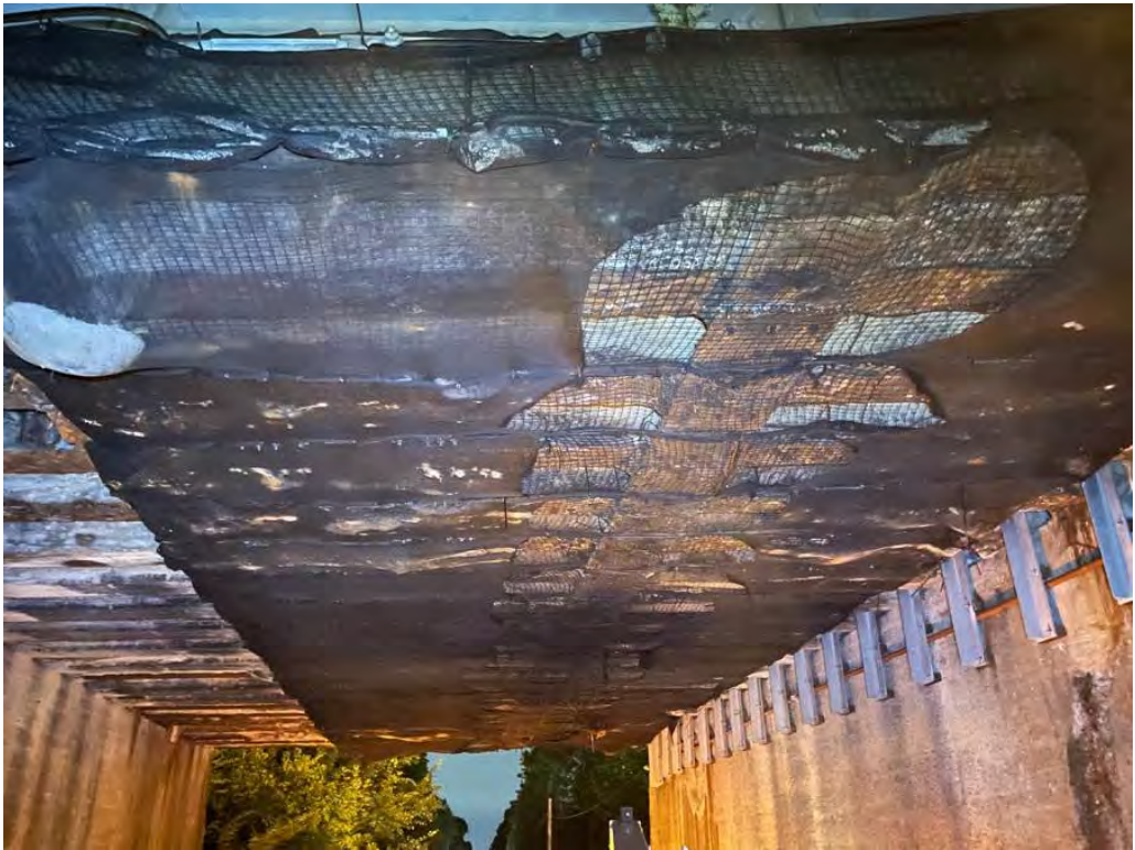
Photo 3: Two layers of netting installed below the bridge, note the bottom layer is torn in several places between west and east fascia beams (view looking east)
