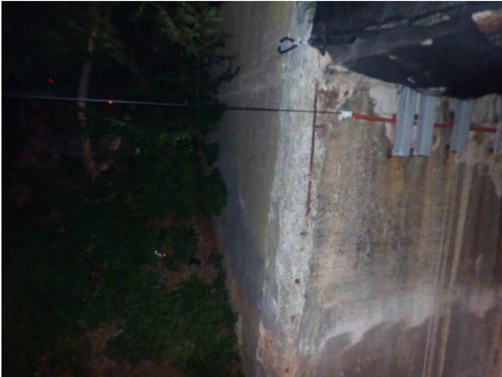
Photo 18: South breastwall at the east end, spalled, full-height x 4-1/2' W x 6" D with exposed rusted rebar
