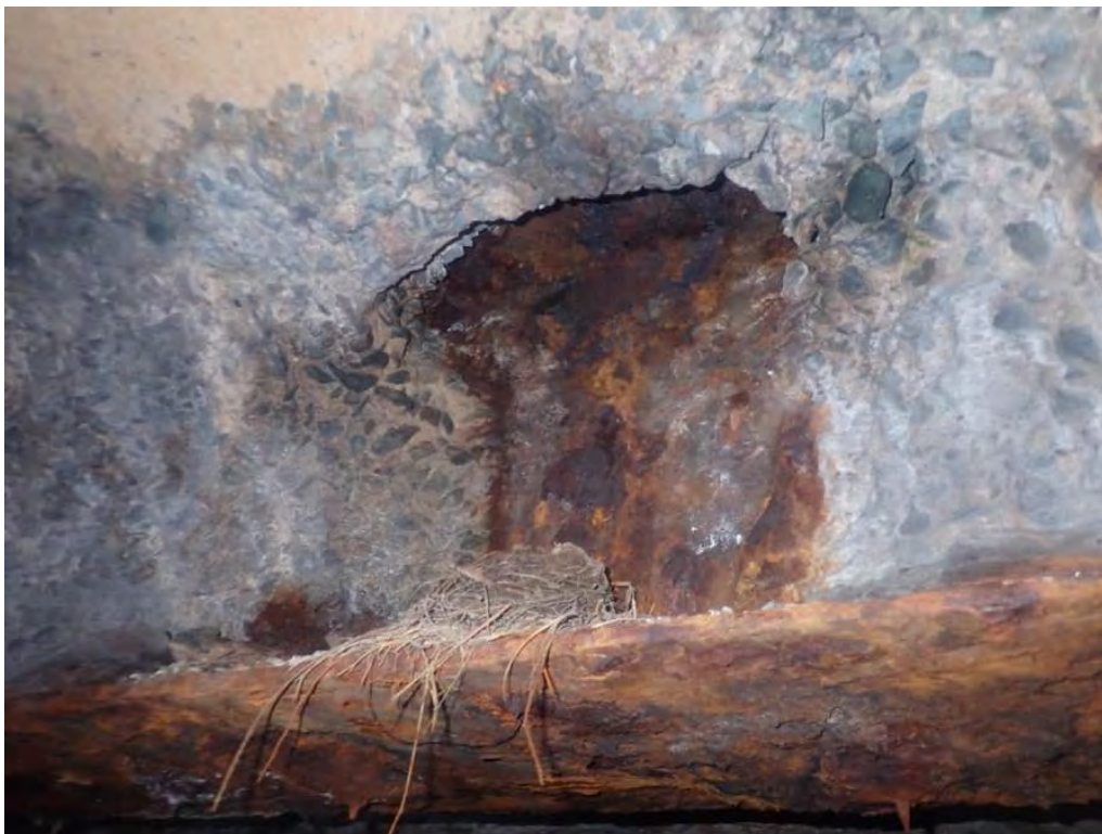
Photo 10: Beam #4, west face spalled with steel web exposed and part of top flange exposed 8' from the north abutment
