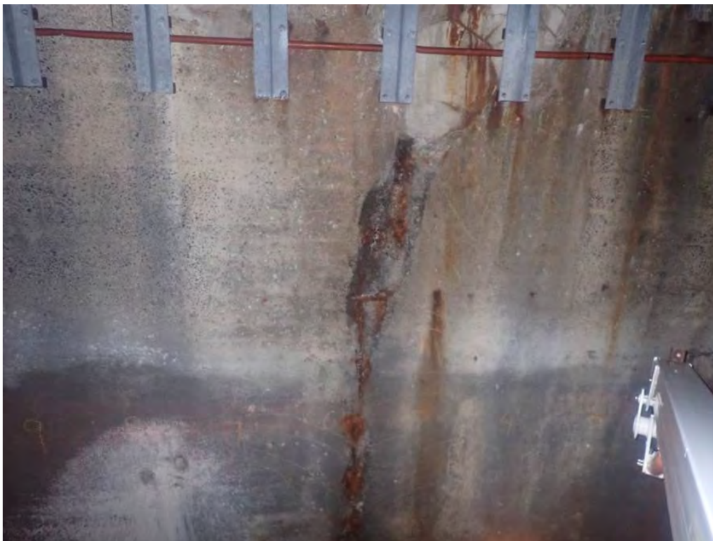
Photo 15: South breastwall between beams #4 and #7, heavy spalling and adjacent hollow concrete with repair at the top 4'
