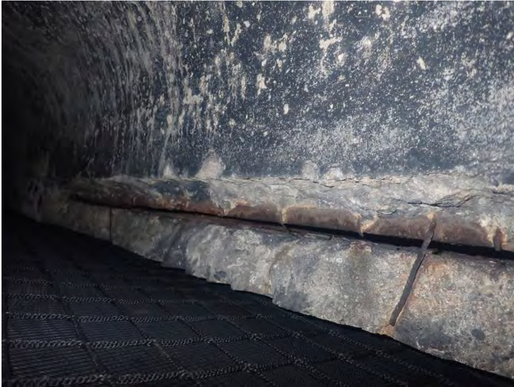
Photo 11: Beam #14, east face, bottom edge of bottom flange spalled with the bottom flange partially exposed at south abutment
