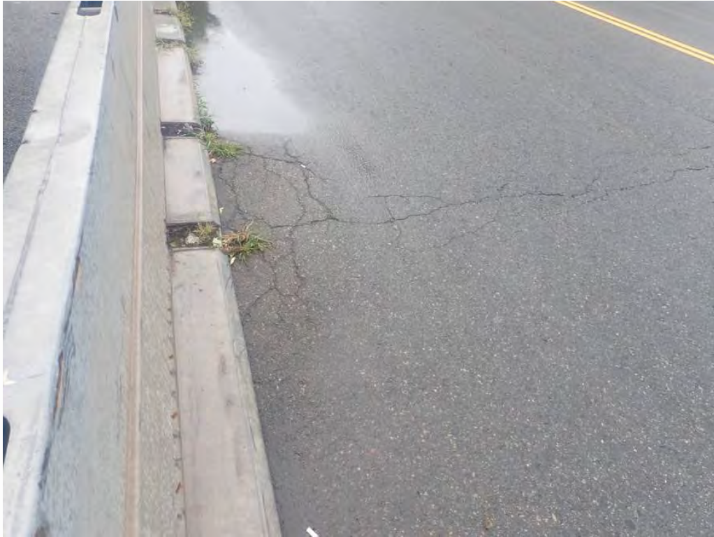
Photo 1: Area of heavy map cracking at the north abutment adjacent to the east railing
