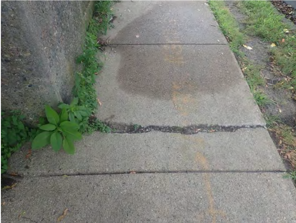
Photo 7: Northeast approach sidewalk has heavy transverse crack in the seventh panel
