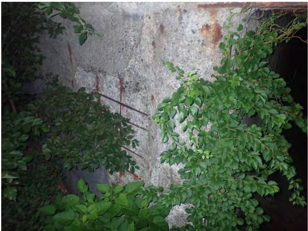
Photo 19: North breastwall and northwest wingwall, heavy spalling
