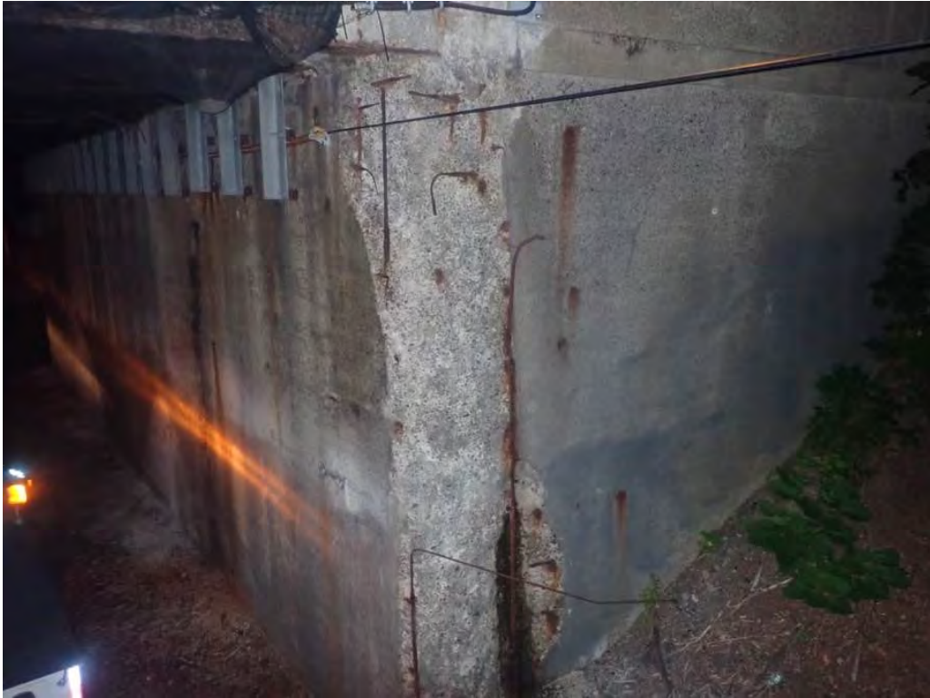
Photo 13: South breastwall, west end, heavy spalling full-height
