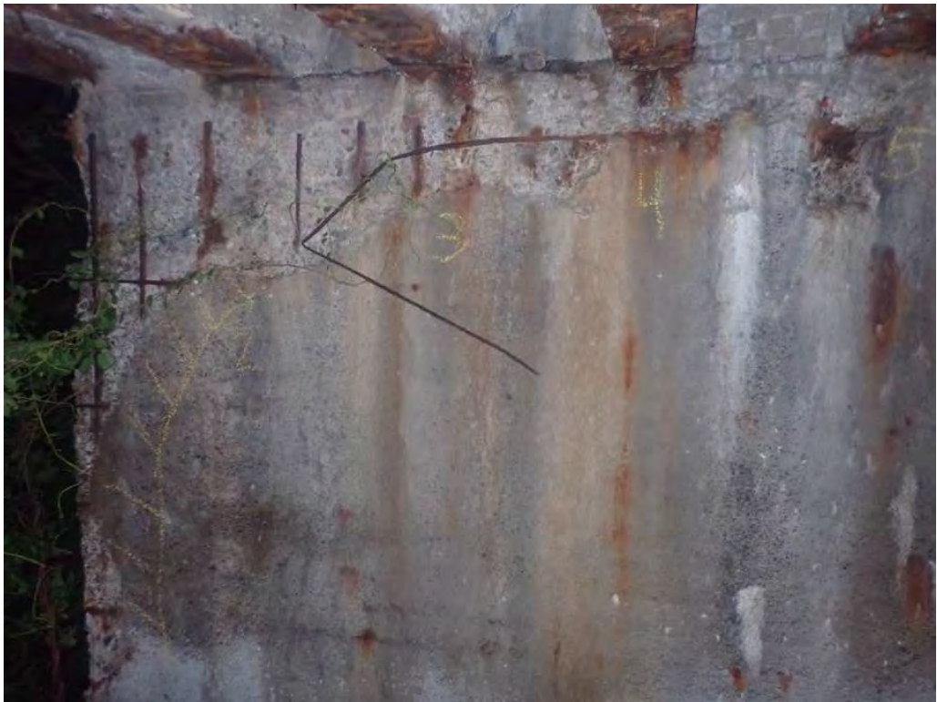
Photo 20: North breastwall, spall at the top below beams #1 to #5, 10' W x 2' H x 3" D with exposed rusted rebar
