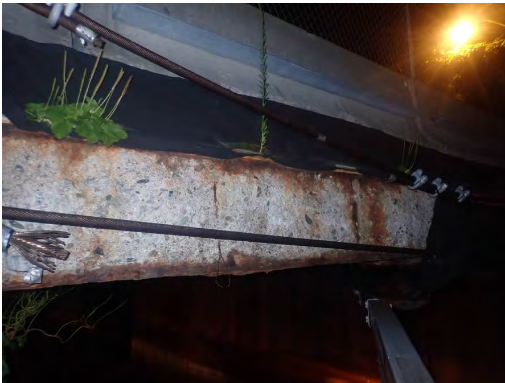
Photo 9: Close up of Beam #1, west fascia beam, with heavy spalling/scaling concrete. Separation between concrete and top flange
