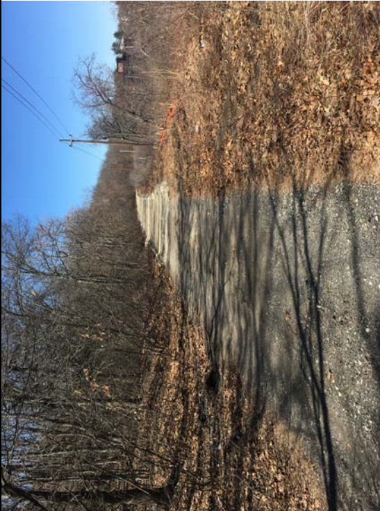
Photo 1: Boundary between Lawrence and Methuen. Rail trail construction ongoing on Methuen side of project. (looking north).
