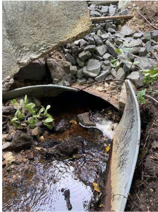
Photo 2: Current upstream elevation. Culvert barrel has been crushed at inlet leaving only about 12" of available vertical clearance for flow. 09/17/2021
