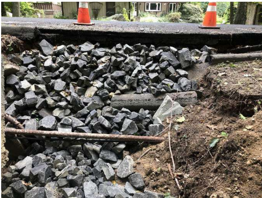
Photo 4: Approach roadway has been compromised due to failed culvert. Erosion has exposed underground utilities and undermined roadway pavement. Temporary riprap has been placed on embankment to help prevent further erosion. 09/17/2021
