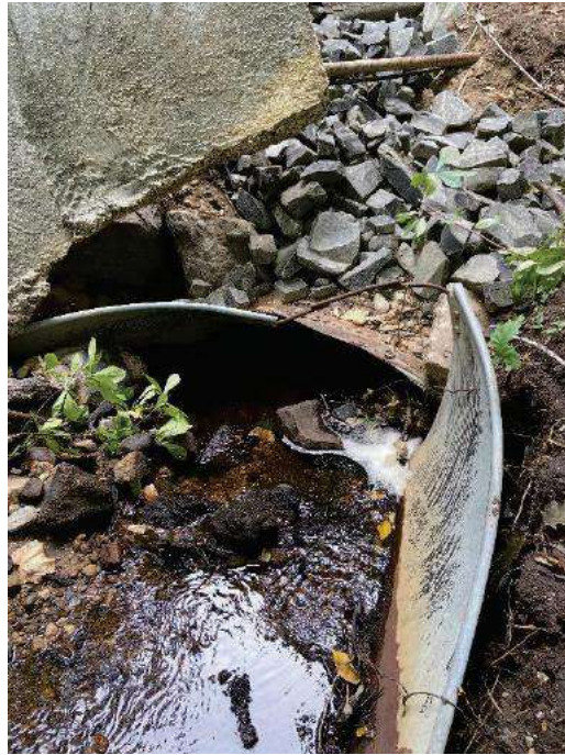
Photo 2: Current upstream elevation. Culvert barrel has been crushed at inlet leaving only about 12" of available vertical clearance for flow. 09/17/2021
