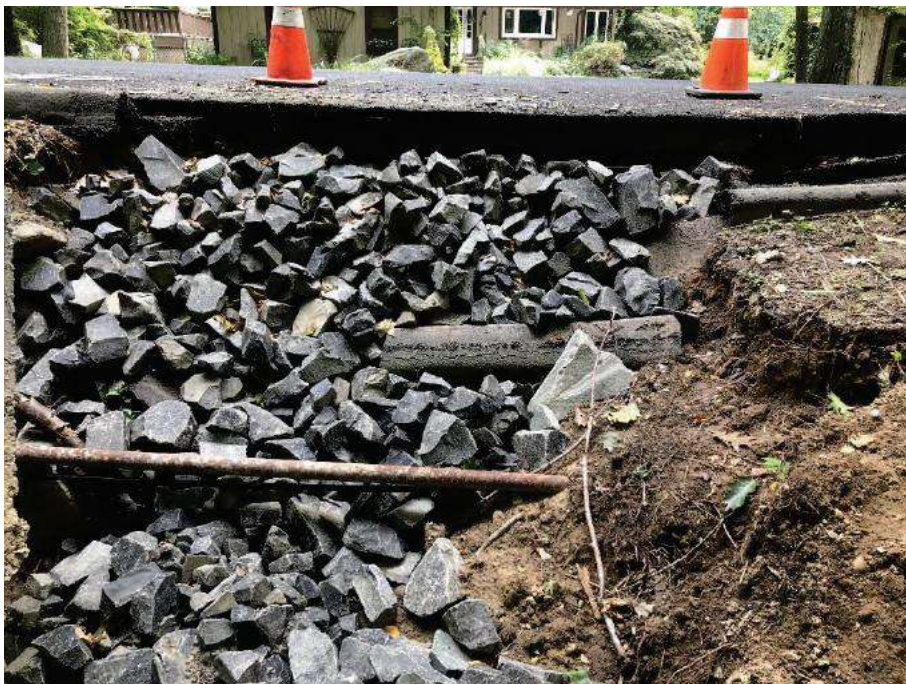
Photo 4: Approach roadway has been compromised due to failed culvert. Erosion has exposed underground utilities and undermined roadway pavement. Temporary riprap has been placed on embankment to help prevent further erosion. 09/17/2021
