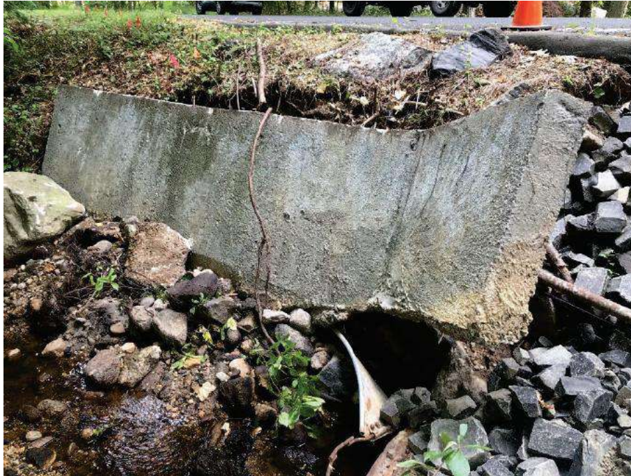
Photo 3: Wingwall collapsed and was originally found on top of crushed barrel. The Town pulled the wingwall back and placed it to help stabilize eroded embankment. 09/17/2021
