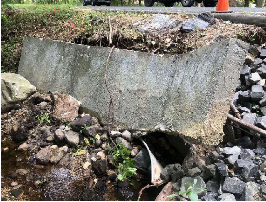
Photo 3: Wingwall collapsed and was originally found on top of crushed barrel. The Town pulled the wingwall back and placed it to help stabilize eroded embankment. 09/17/2021
