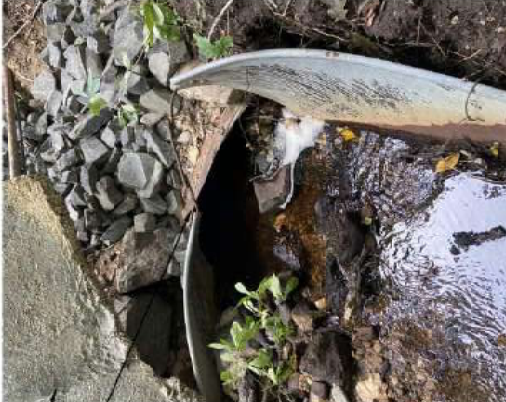
Failed Concrete Wing Wall Crushed 54"x39" CMP Arch (Approx. 48"x12" At Inlet)
