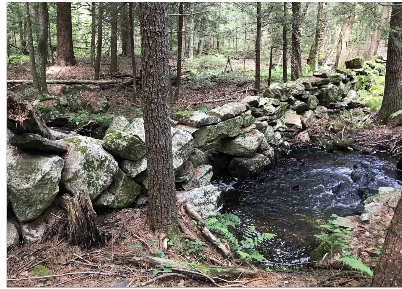
PHOTO NO. 1 EXISTING STONE WALL TO BE PROTECTED AND TO REMAIN INTACT
