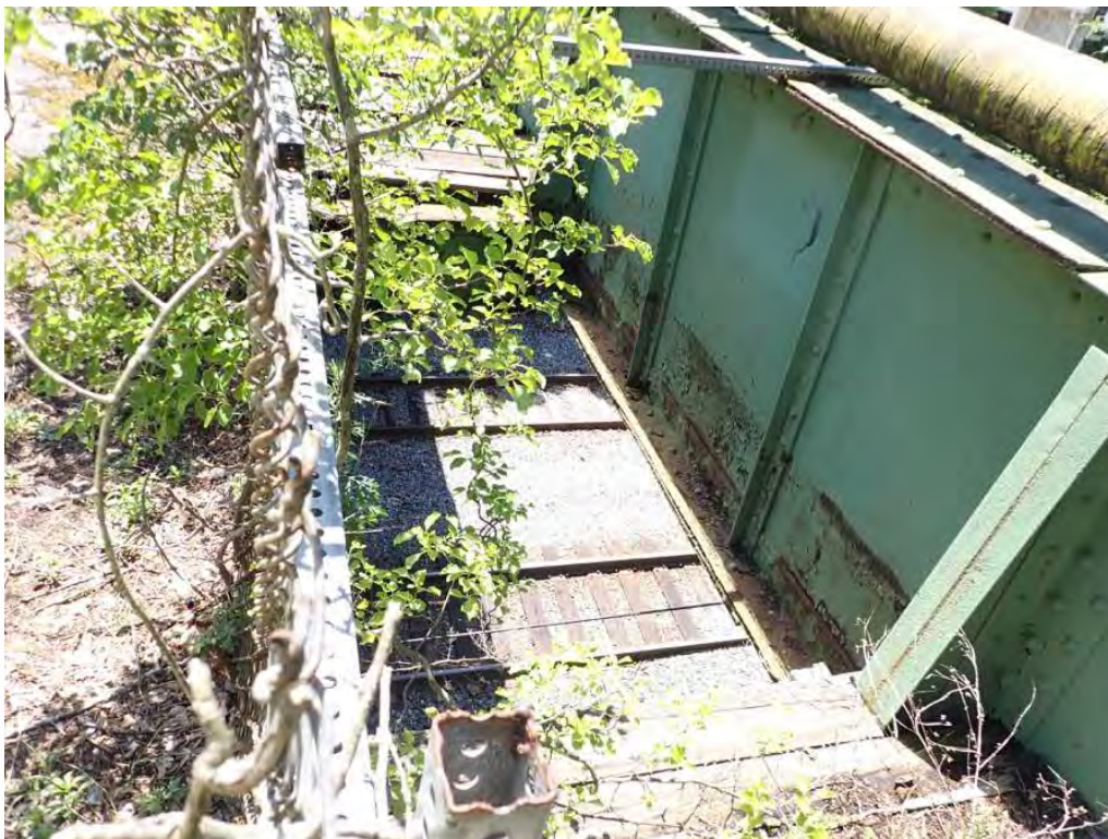
Photo 5: West sidewalk, missing section.
