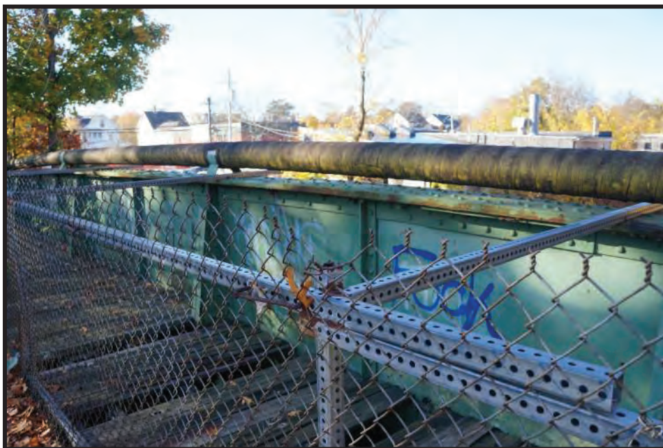
Photo 8: Gas utility attached to the top of the West through girder, looking Southwest.
