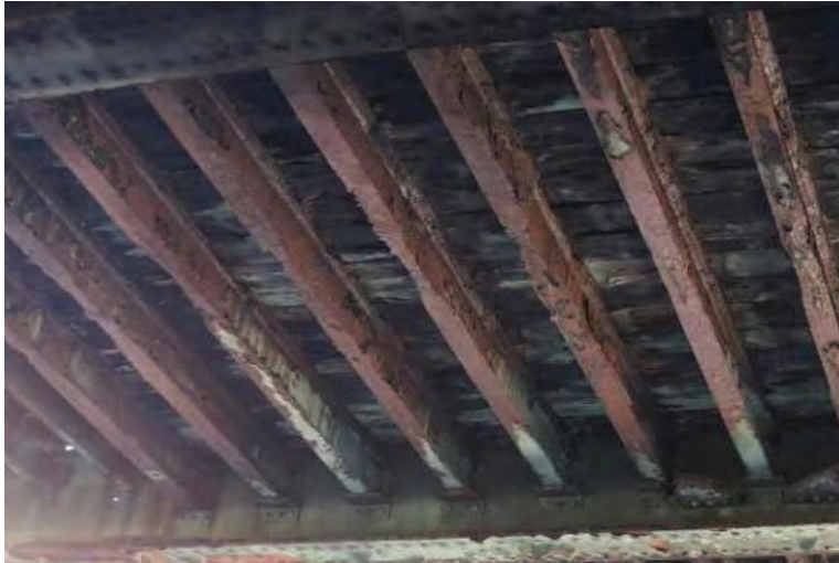
Typical condition of the stringers, showing significant section loss to the bottom flanges.
