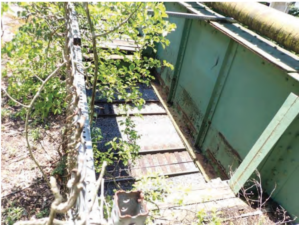
Photo 5: West sidewalk, missing section.
