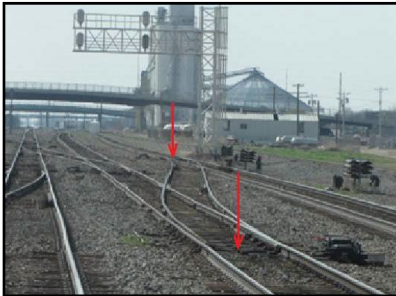
Figure 16 – Point of Switch – Crossover Switches
