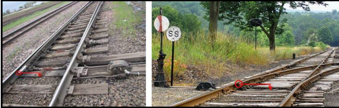
Figure 15 – Point of Switch – Spring Switch
