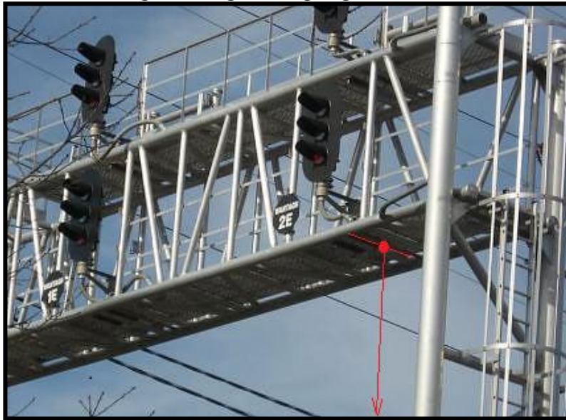
Figure 9 – Signal Bridge Signal Location
