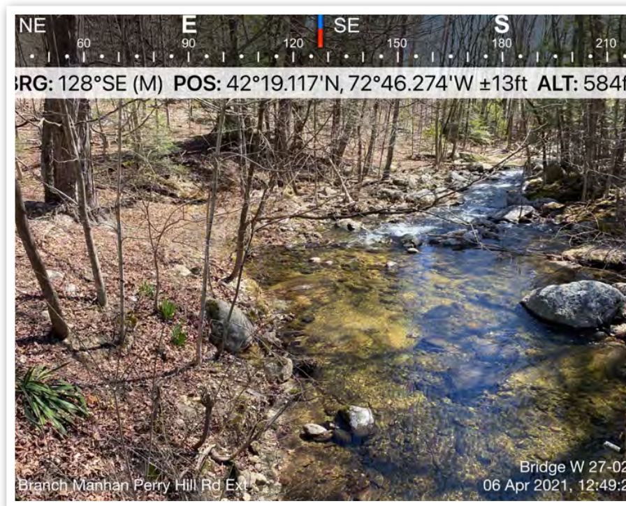
April 06, 2021 View from the bridge over the N. Branch of the Manhan looking downstream at the east bank and due southeast.
