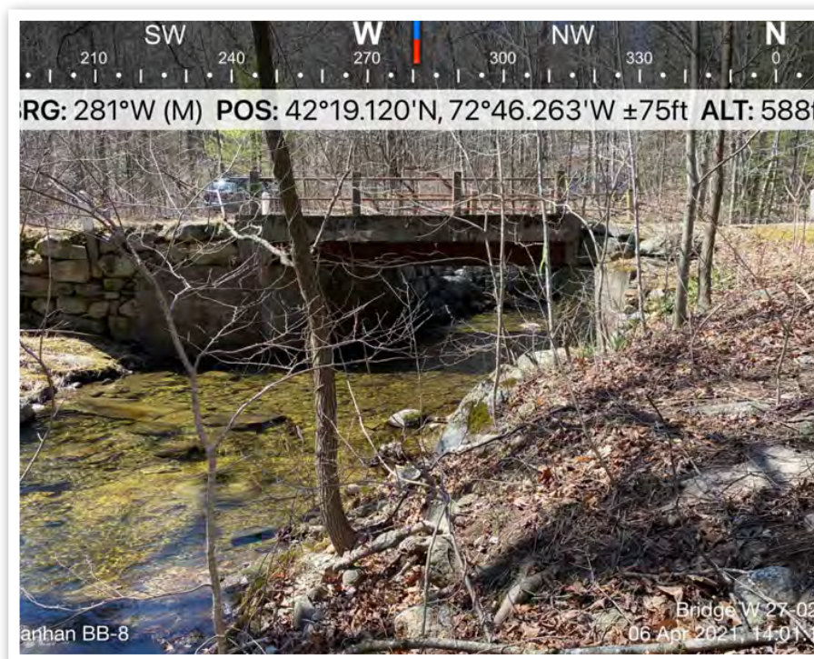
April 06, 2021 Looking stream at the bridge from the downstream side with the eastern bank on viewers right.
