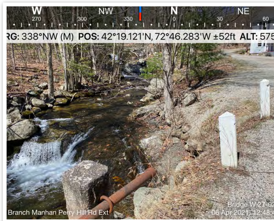
April 06, 2021 View from the bridge over the N. Branch of the Manhan looking upstream at the east bank and due NNW.
