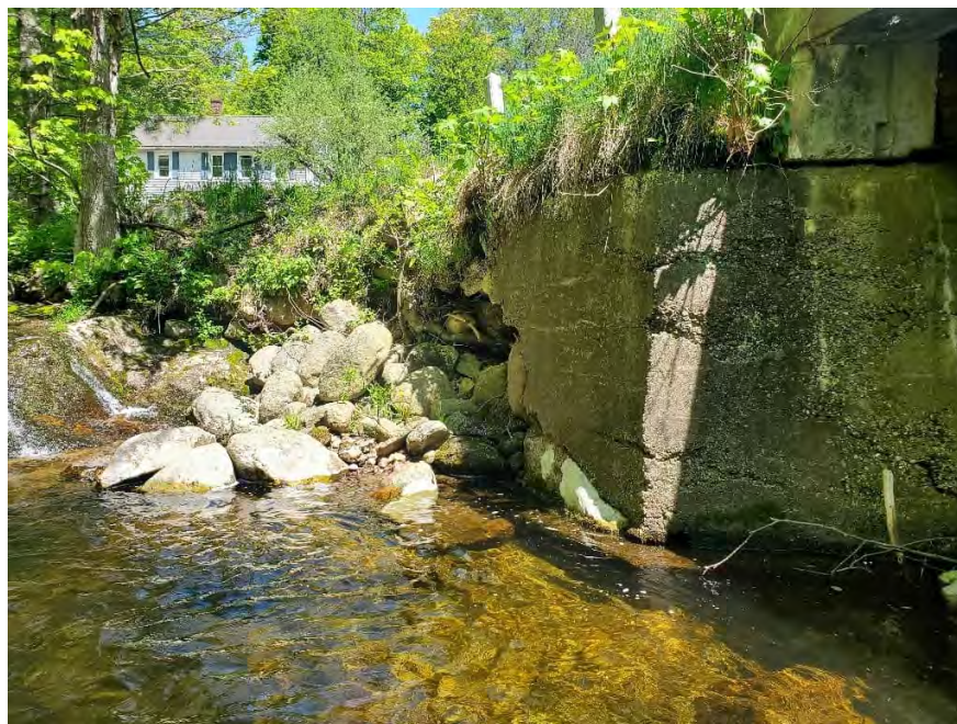
Figure 7: Left Bank Failure Upstream of Bridge
