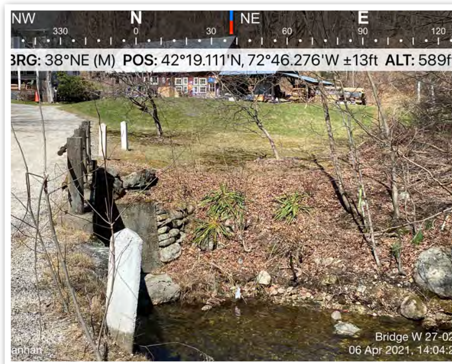
April 06, 2021 View of the downstream side of the bridge looking due northeast at the eastern bank.
