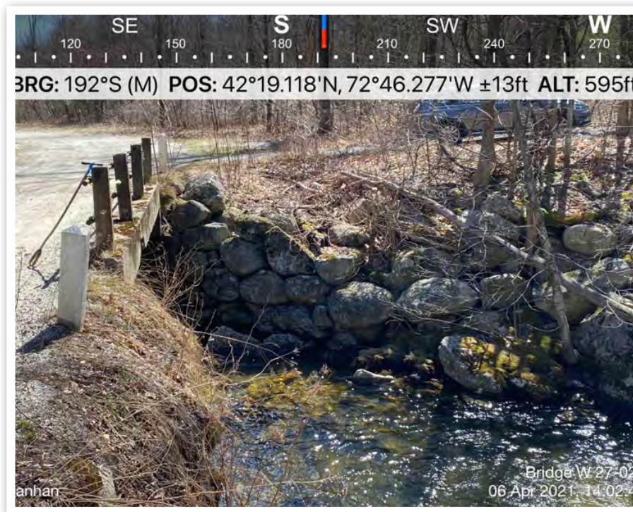
April 06, 2021 View of the upstream side of the bridge looking due southwest at the western bank.
