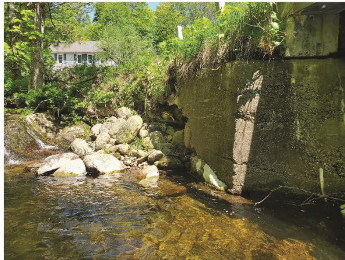
Figure 7: Left Bank Failure Upstream of Bridge
