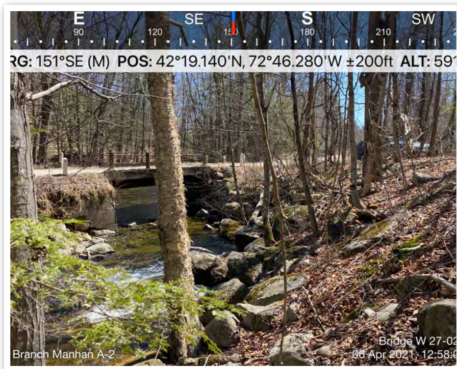
April 06, 2021 View from upstream of the bridge over the N. Branch of the Manhan looking downstream at the west bank and due southeast.
