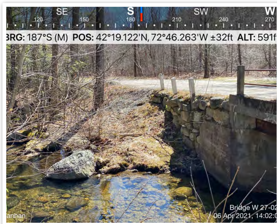
April 06, 2021 View of the downstream side of the bridge looking due southwest at the western bank.
