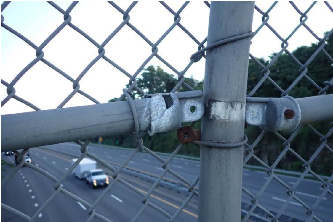
Photo 20: Typical condition of some of the frame connections.
