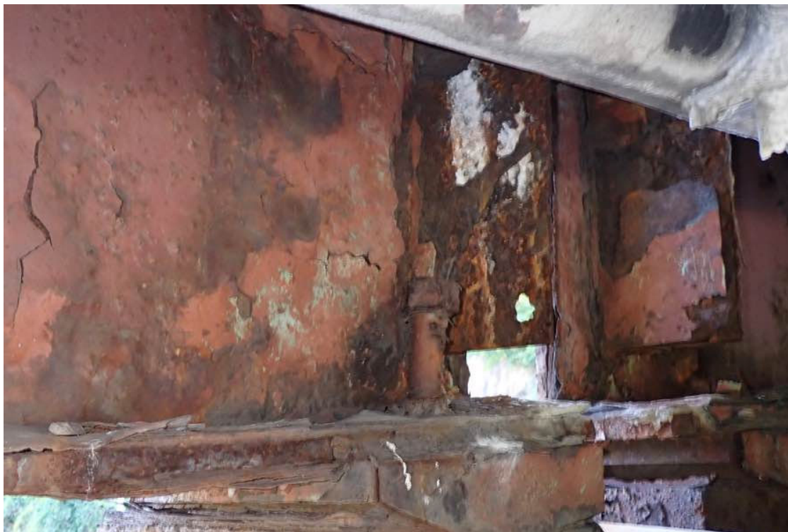
Photo 45: End diaphragm connection plate at the west end of beam S1 (pier end).
