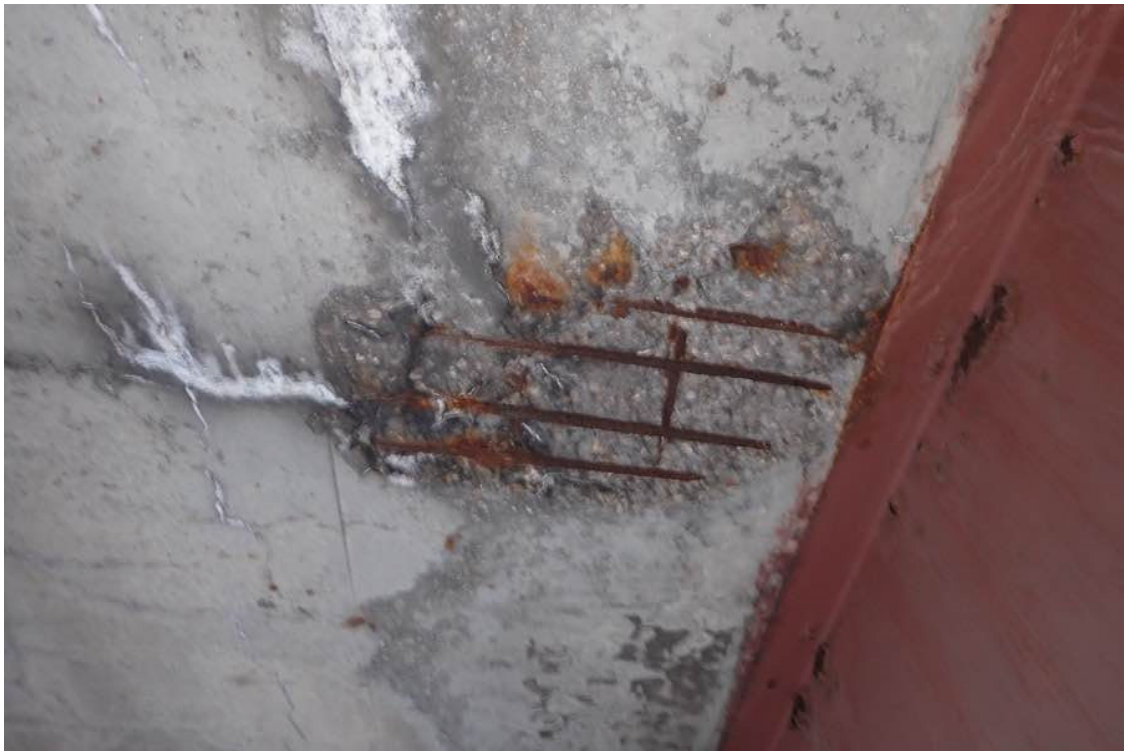
Photo 12: Spall in bay 3 of span 1 over the middle travel lane.
