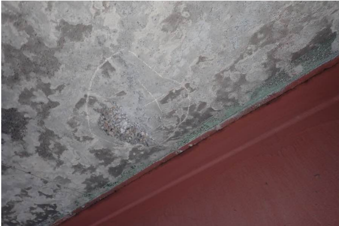
Photo 11: Spall in bay 2 of span 1 over the ramp lane.
