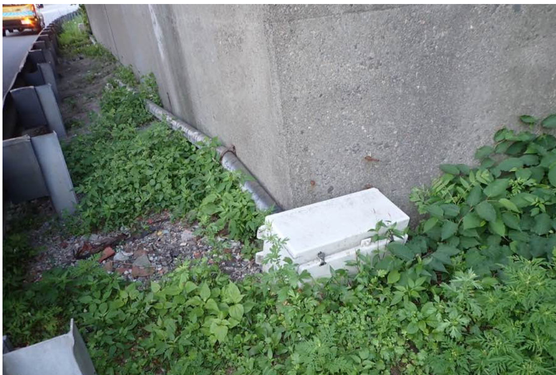
Photo 22: Utility box laying on the ground at the west abutment.
