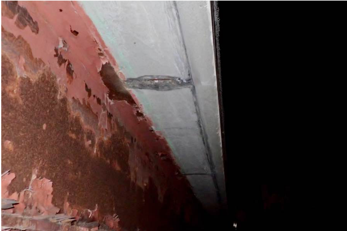
Photo 5: South deck fascia in span 2, spall over I-290 EB.
