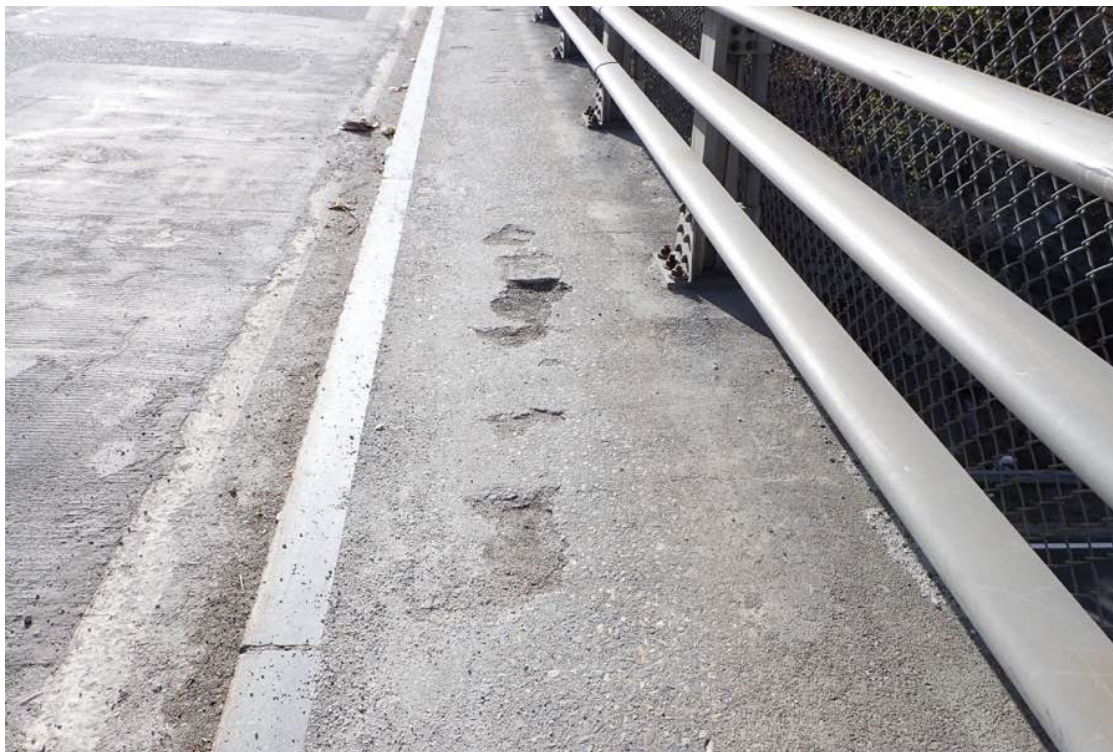
Photo 7: Typical deterioration to the sidewalks. North sidewalk shown.
