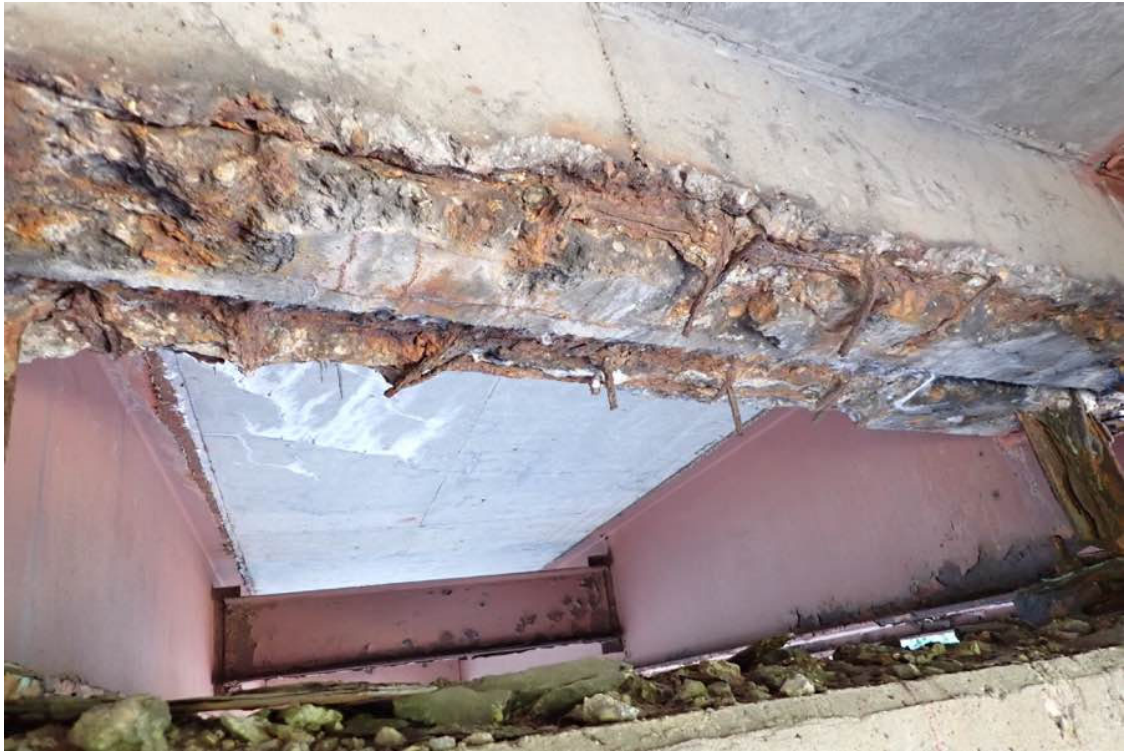
Photo 47: Typical condition of the end diaphragms over the pier.
