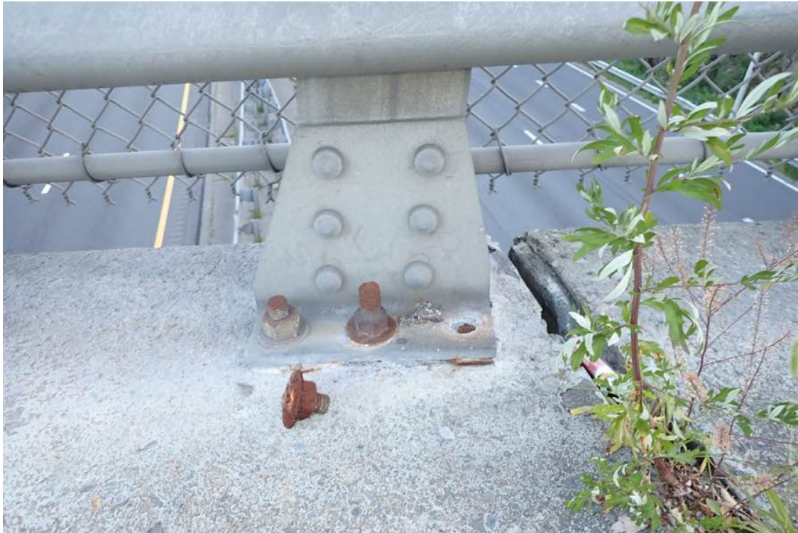
Photo 19: North railing at the 9th post from the west (pier joint location).
