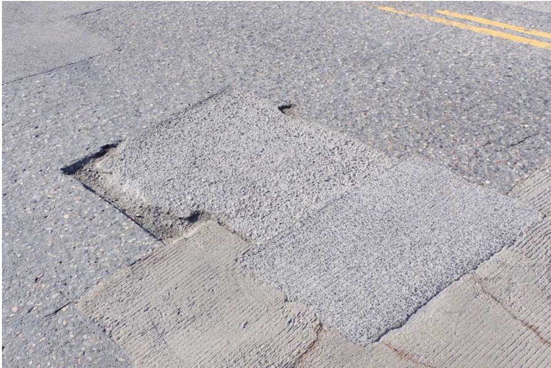
Photo 3: Scale to a repair patch in the westbound lane, span 1.
