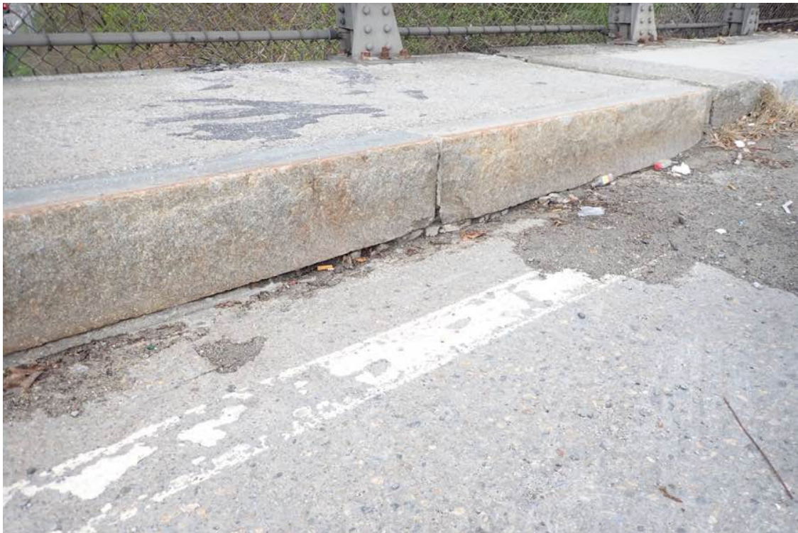
Photo 6: Curb pointing deterioration.
