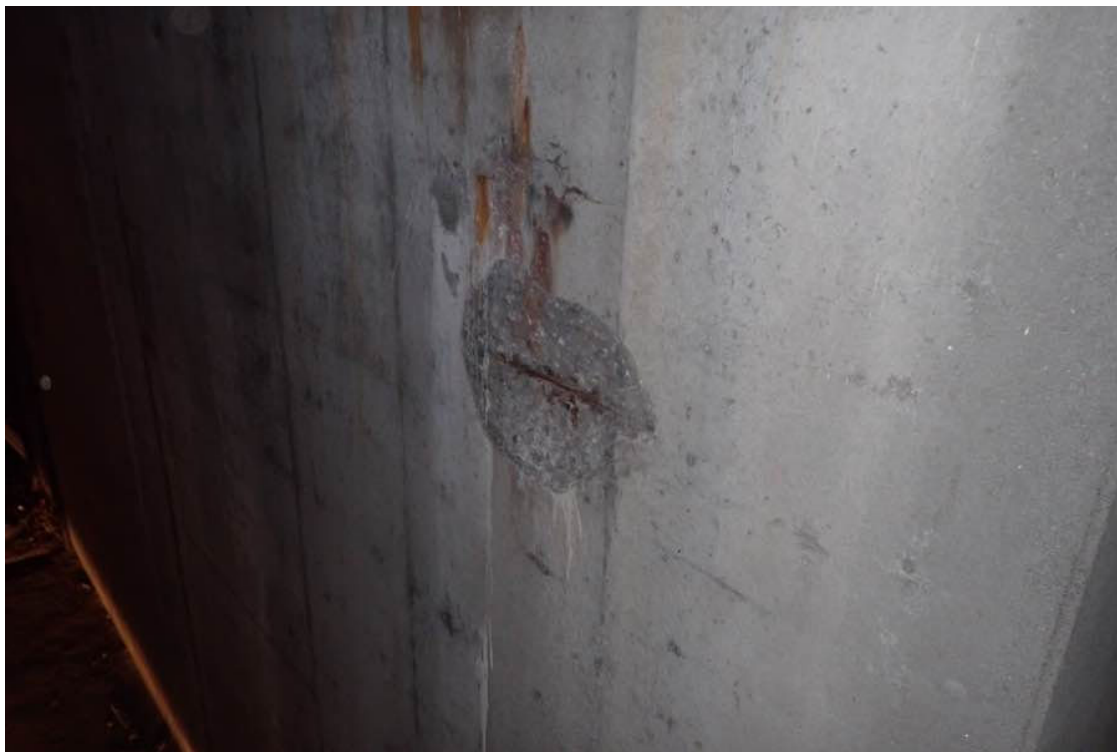
Photo 47: Spall to the east backwall below bay 6.
