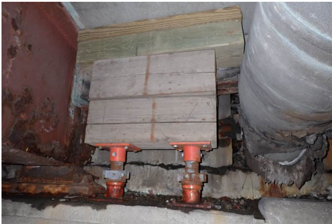
Photo 35: Screw jacks at beam 7, west abutment.
