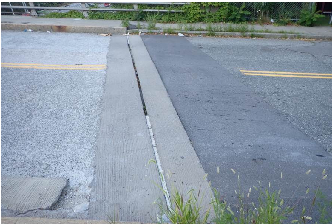
Photo 3: West end of the wearing surface in span 1 and approach to deck transition.
