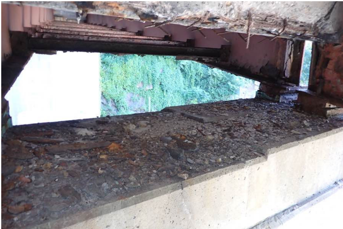
Photo 58: Debris on top of the pier cap in bay #5.
