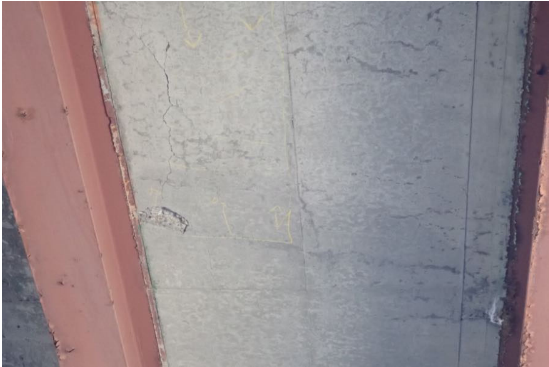
Photo 15: Delamination cracking in bay 4 over the middle travel lane.
