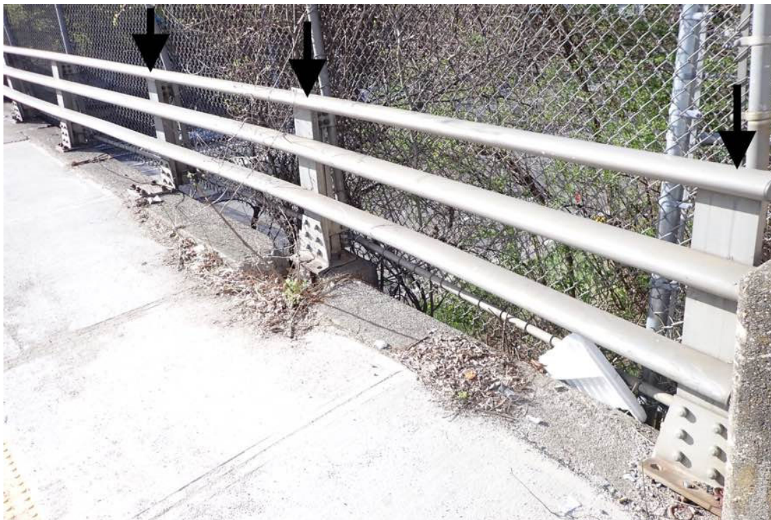
Photo 8: Collision damage to the south AL-3 railing at the west end.
