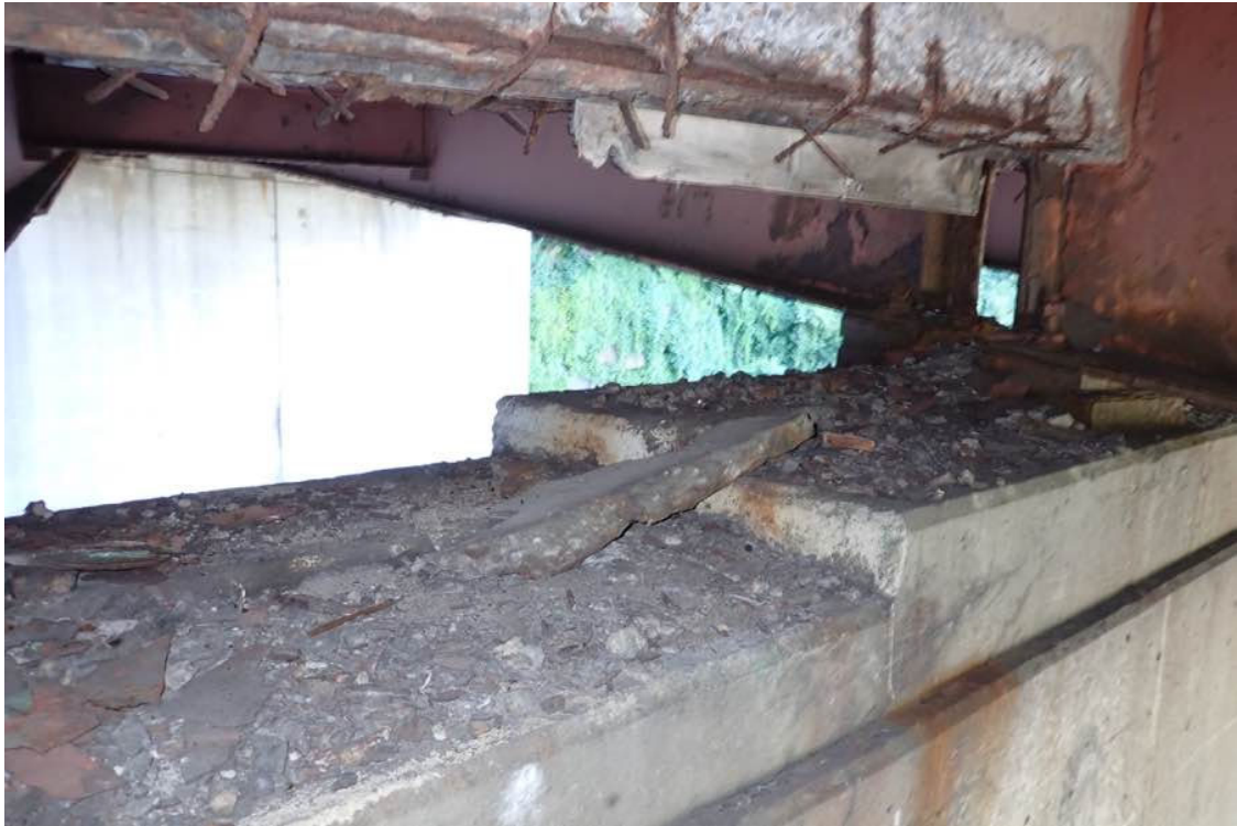
Photo 59: Debris on top of the pier cap in bay #2.
