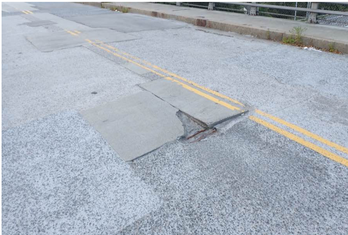
Photo 5: Spall to the wearing surface in WB lane in span 1.
