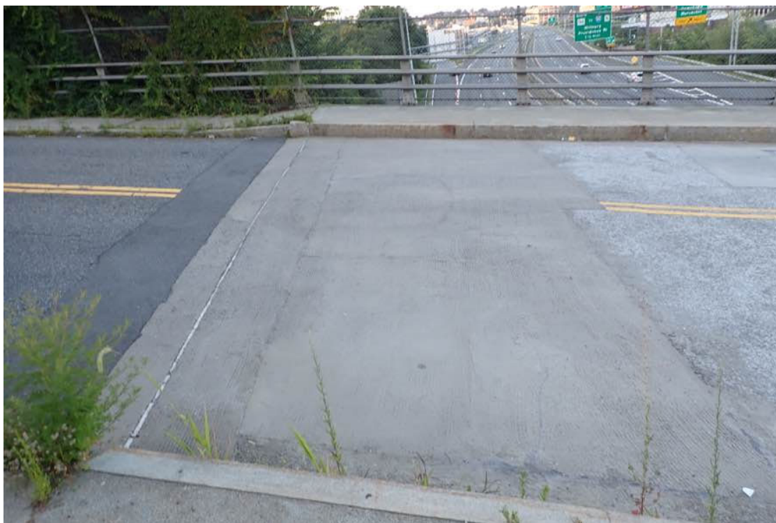
Photo 4: East end of the deck in span 2 and approach to deck transition.
