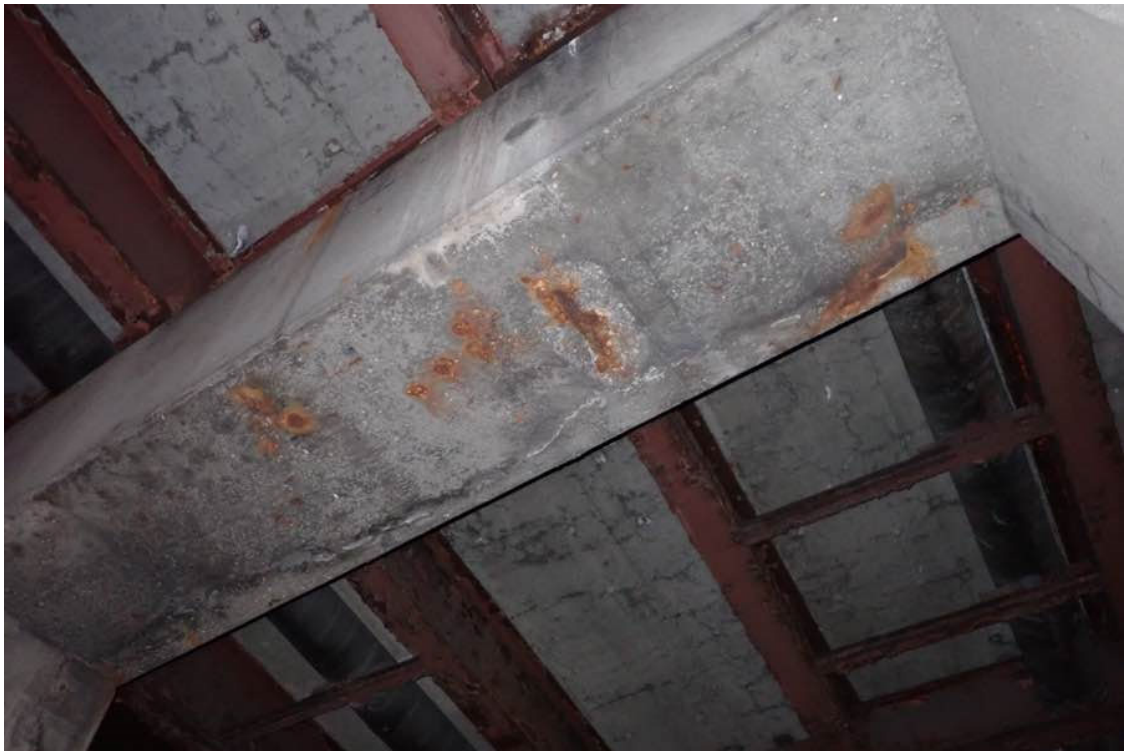
Photo 50: Spall on the underside of the pier cap between columns 2 and 3.
