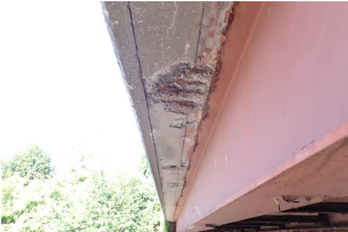
Photo 10: South deck fascia in span 1 over the left and middle travel lanes.
