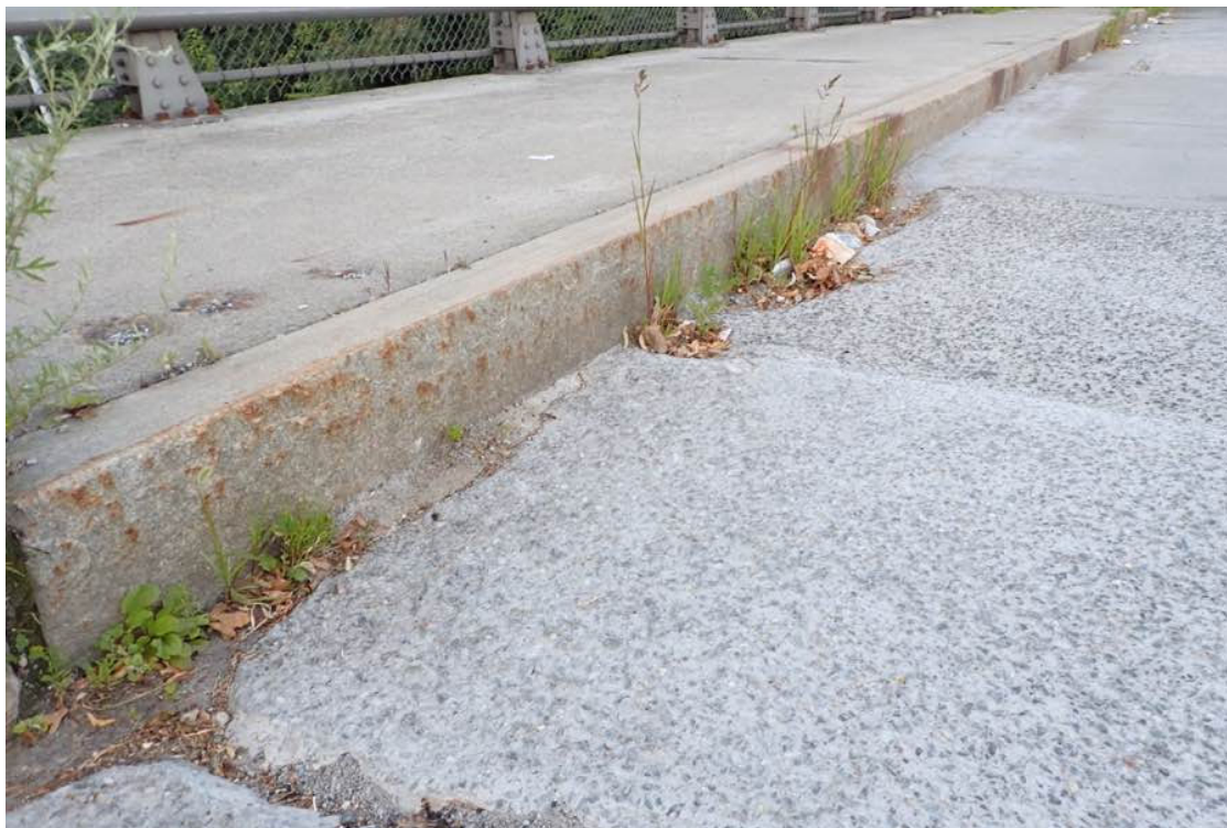
Photo 6: Scale areas to the repair patches along the south curb in span 1 filled with dirt and vegetation.
