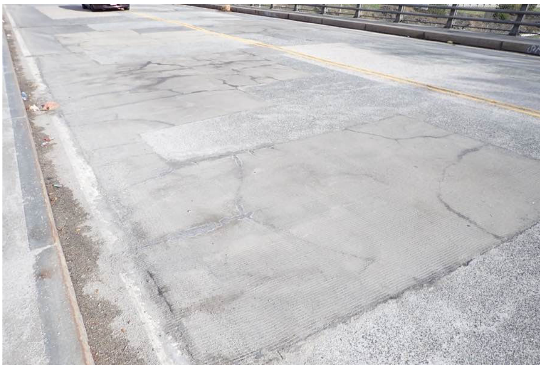
Photo 2: Typical condition of the rapid set concrete patches.
