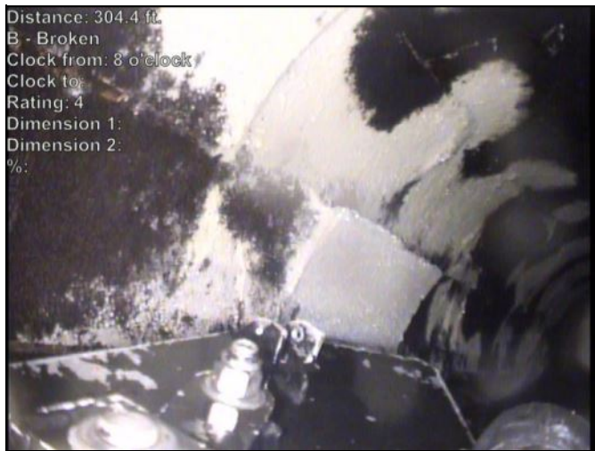
Distance: 304.4 ft. B - Broken Clock from: 8 o'clock Clock to: Rating: 4 Dimension 1: Dimension 2: %: Photo: 79A-799-20230502-094355-101037.JPG At: 304.433 ft. B - Broken 8/. Joint: No
