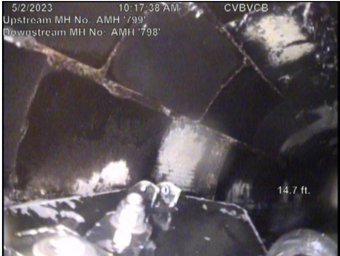
Photo: 799-798-20230502-101533-101734.JPG At: 13.11 ft. 8/. B - Broken Joint: No
