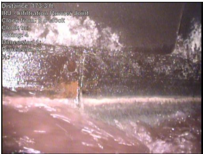
Distance: 173.3 ft. IRJ - Infiltration Runner Joint Clock from: 8 o'clock Clock to: Rating: 4 Dimension 1: Dimension 2: %: Photo: 795-794-20230503-092055-094551.JPG At: 173.333 ft. IRJ - Infiltration Runner Joint 8/. Joint: Yes
