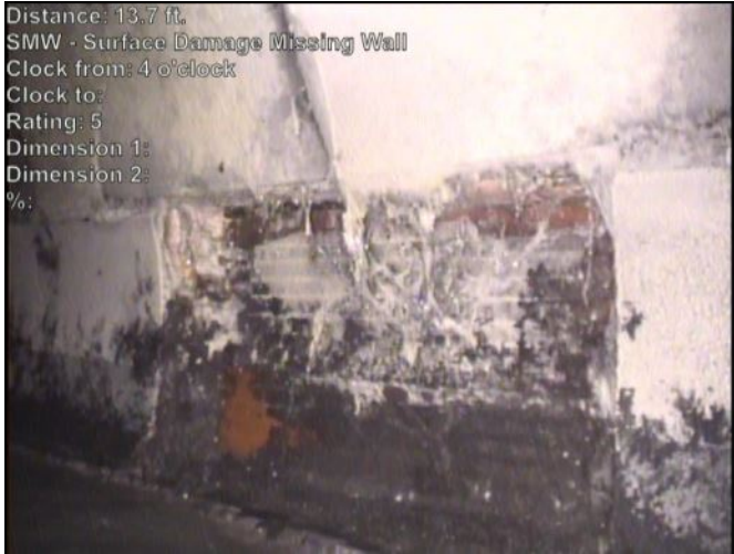
Photo: 797-796-20230503-083917-084200.JPG At: 13.71 ft. 4/. SMW - Surface Damage Missing Wall Joint: No
