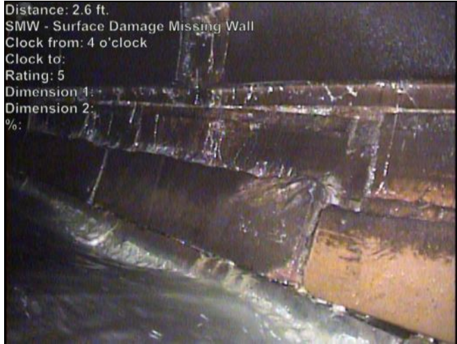
Photo: J-8102-7D8-20230503-130327-130415.JPG At: 2.602 ft. 4/. SMW - Surface Damage Missing Wall Joint: No
