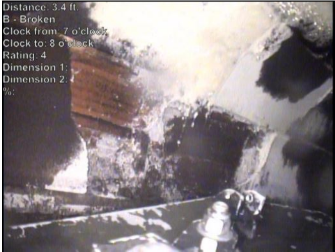
Photo: 799-798-20230502-101533-101625.JPG At: 3.403 ft. 7/8 B - Broken Joint: No
