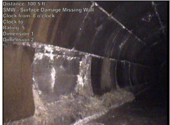
Photo: 795-794-20230503-092055-093810.JPG At: 100.477 ft. SMW - Surface Damage Missing Wall 8/. Joint: No
