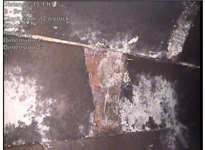
Photo: J-8102-7D8-20230503-130327-130507.JPG At: 15.412 ft. B - Broken 12/. Joint: No
