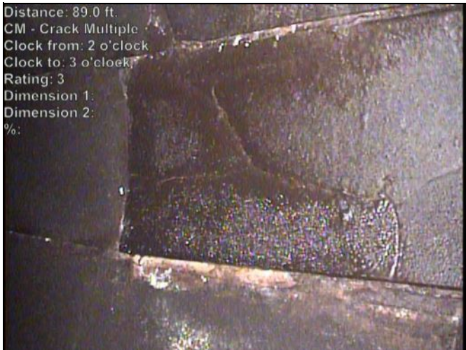
Photo: 792-791-20230503-122735-123141.JPG At: 88.968 ft. CM - Crack Multiple 2/3 Joint: No
