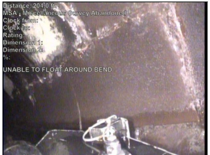
Distance: 204.0 ft. MSA - Miscellaneous Survey Abandoned Clock from: Clock to: Rating: Dimension 1: Dimension 2: %: UNABLE TO FLOAT AROUND BEND Photo: 798-797-20230502-103631-123735.JPG At: 203.956 ft. MSA - Miscellaneous Survey Abandoned Joint: No UNABLE TO FLOAT AROUND BEND
