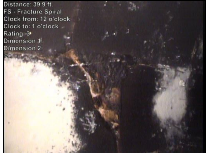
Photo: 798-797-20230502-103631-104032.JPG At: 39.931 ft. FS - Fracture Spiral 12/1 Joint: No
