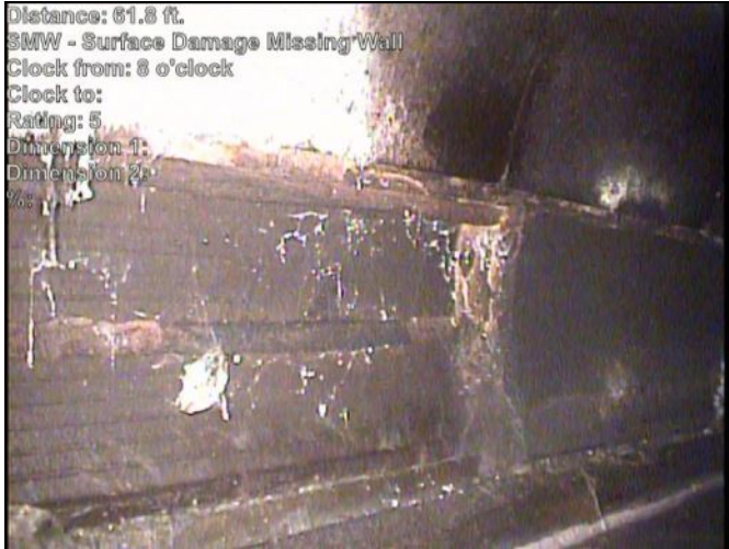
Photo: 792-791-20230503-122735-123022.JPG At: 61.847 ft. 8/. SMW - Surface Damage Missing Wall Joint: No
