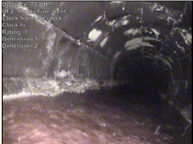
Photo: 795-794-20230503-092055-092638.JPG At: 75.758 ft. 8/. RFJ - Roots Fine Joint Joint: Yes
