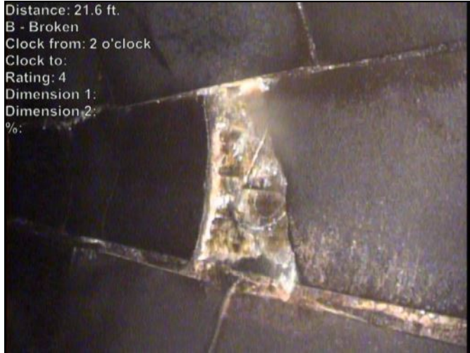
Photo: 795-794-20230503-092055-092244.JPG At: 21.617 ft. 2/. B - Broken Joint: No
