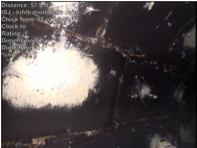
Photo: 798-797-20230502-103631-104309.JPG At: 57.944 ft. ISJ - Infiltration Stain Joint 12/. Joint: Yes
