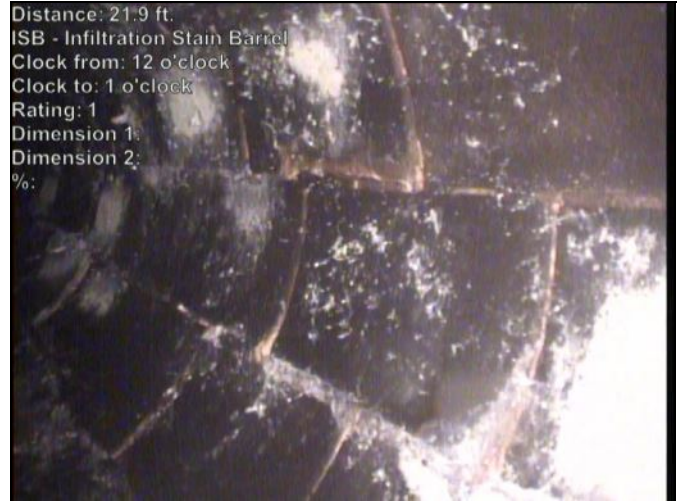
Photo: 798-797-20230503-081307-082847.JPG At: 21.917 ft. ISB - Infiltration Stain Barrel 12/1 Joint: No
