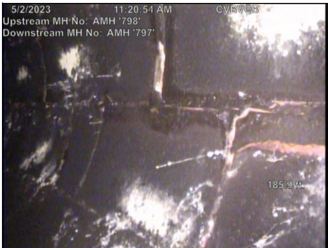
5/2/2023 11:20:54 AM CVBVGB Upstream MH No: AMH '798' Downstream MH No: AMH '797' 185.9 ft. Photo: 798-797-20230502-103631-112049.JPG At: 184.942 ft. ISJ - Infiltration Stain Joint 1/. Joint: Yes
