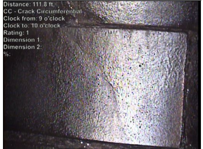
Photo: 793-792-20230503-120748-121131.JPG At: 111.786 ft. CC - Crack Circumferential 9/10 Joint: No
