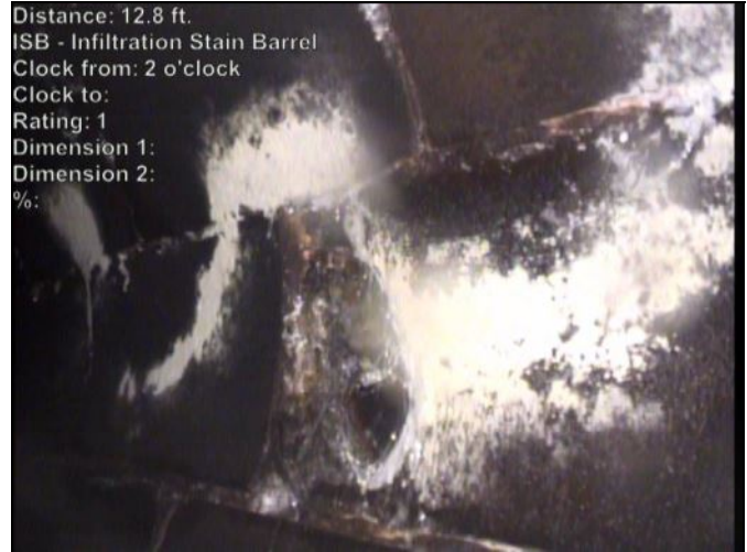
Photo: 799-798-20230502-101533-101713.JPG At: 12.81 ft. 2/. ISB - Infiltration Stain Barrel Joint: No
