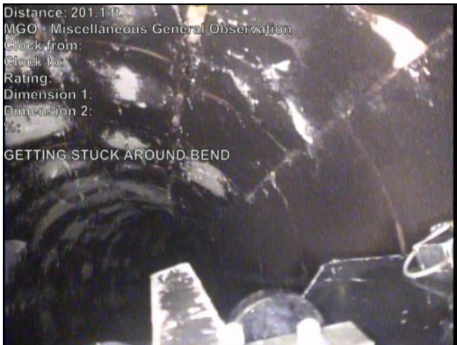
Distance: 201.1 ft. MGO - Miscellaneous General Observation Clock from: Clock to: Rating: Dimension 1: Dimension 2: %: GETTING STUCK AROUND BEND Photo: 798-797-20230502-103631-114256.JPG At: 201.054 ft. MGO - Miscellaneous General Observation Joint: No GETTING STUCK AROUND BEND
