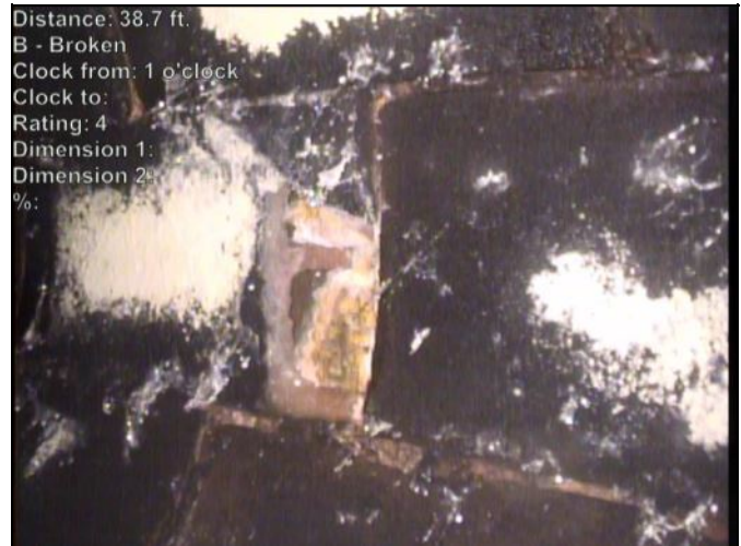
Photo: 798-797-20230503-081307-082951.JPG At: 38.73 ft. 1/. B - Broken Joint: No
