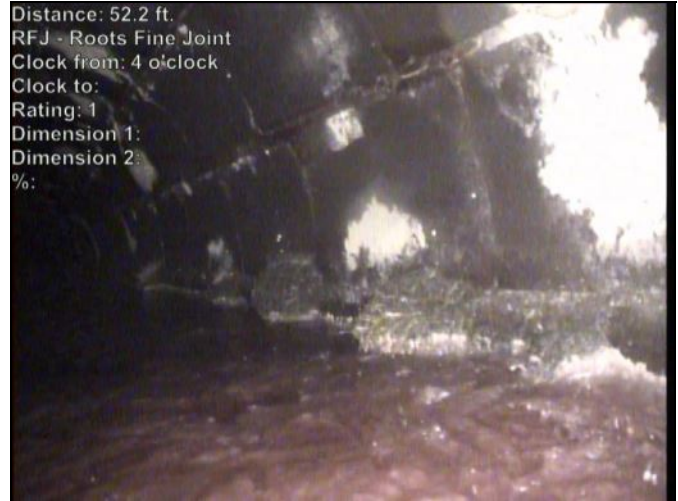
Photo: 795-794-20230503-092055-092451.JPG At: 52.24 ft. 4/. RFJ - Roots Fine Joint Joint: Yes
