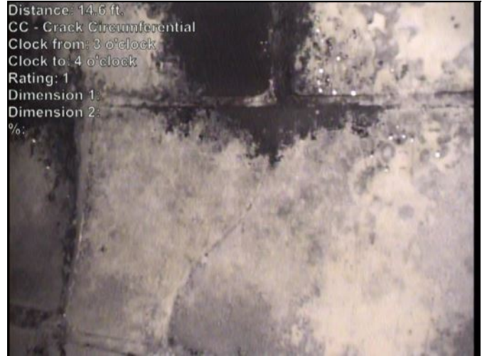
Photo: 797-796-20230503-083917-084251.JPG At: 14.611 ft. CC - Crack Circumferential 3/4 Joint: No
