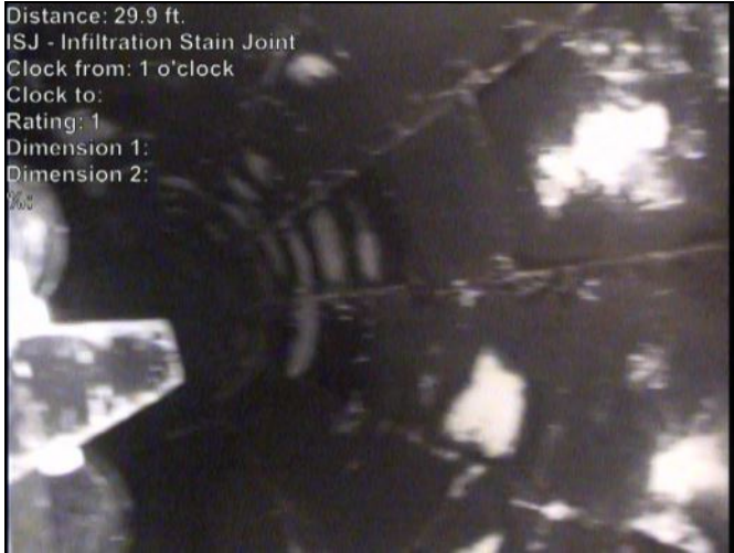
Photo: 798-797-20230502-103631-103835.JPG At: 29.923 ft. 1/. ISJ - Infiltration Stain Joint Joint: Yes
