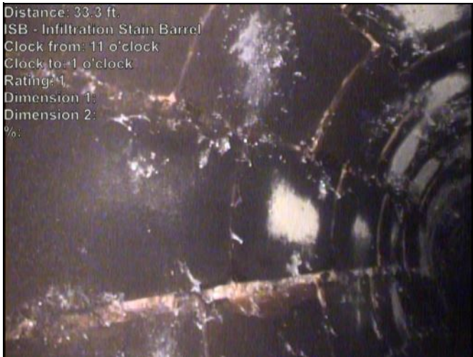
Photo: 798-797-20230503-081307-082924.JPG At: 33.326 ft. ISB - Infiltration Stain Barrel 11/1 Joint: No
