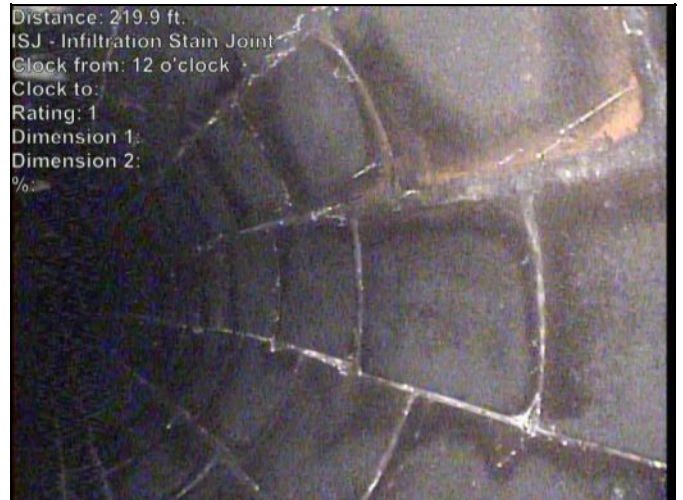
Photo: 793-792-20230503-120748-121450.JPG At: 219.868 ft. ISJ - Infiltration Stain Joint 12/. Joint: Yes
