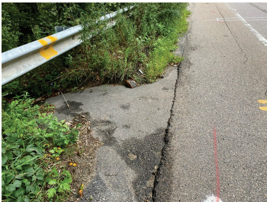
Photo 1. View of paved swale at STA 22+75 directing untreated stormwater runoff onto the hillside embankment and into the Vernal Pool proximate to Wetland Flag #11.
