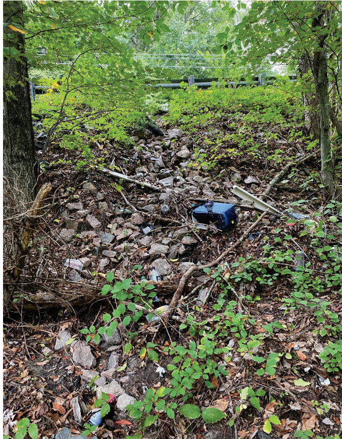
Photo 2. View of steep hillside embankment with rip-rap downgradient of paved swale at STA 22+75. Untreated stormwater runoff flows over the embankment and into the Vernal Pool proximate to Wetland Flag #11. Note erosion of embankment and trash. Sediment accumulation observed at bottom of slope (not pictured).
